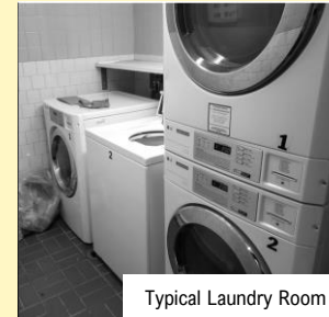
Typical Laundry Room
