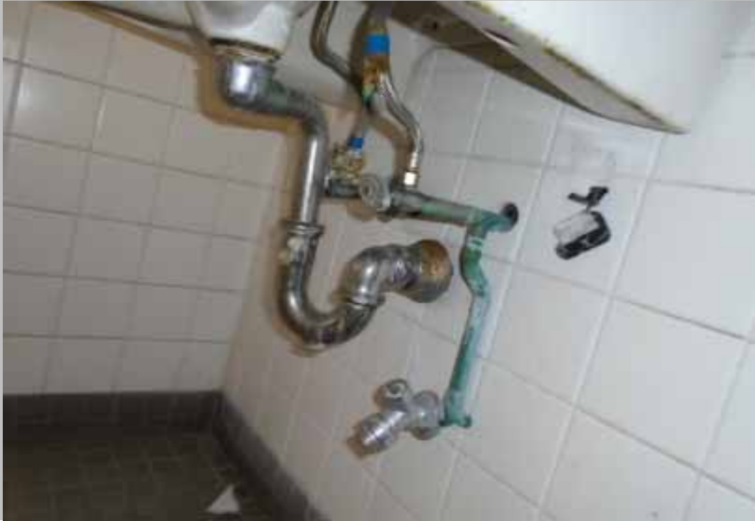
Install Scald and Abrasion Protection at Men's Public Restroom Sink (Critical Repair)
