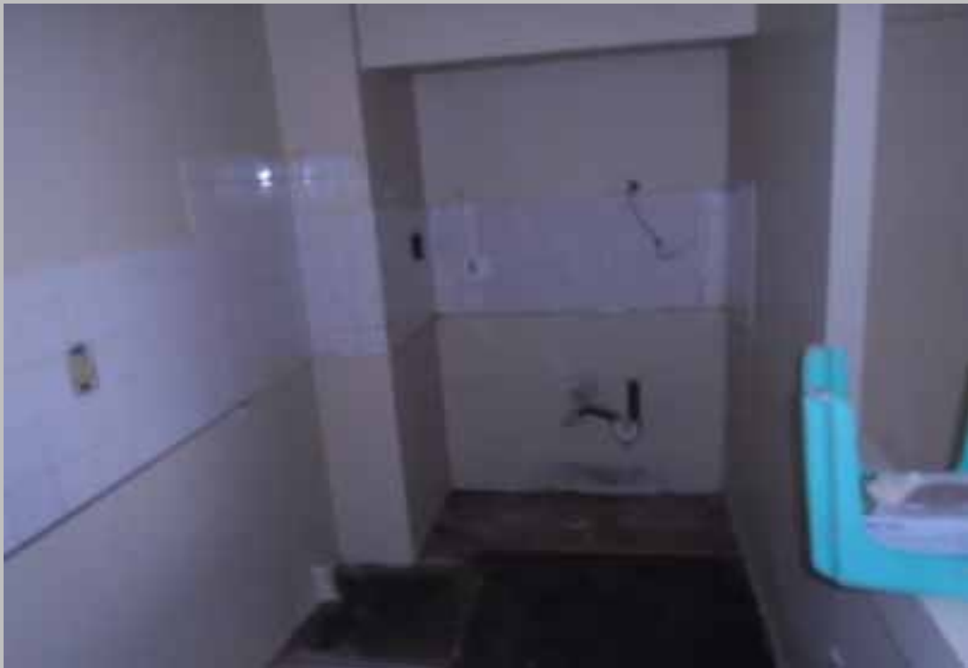
Complete Turn in Unit 607 (Non-Critical Repair)
