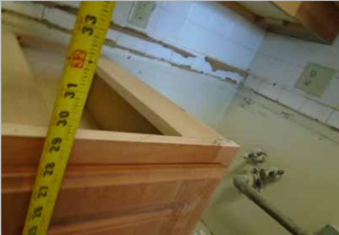
Complete Turn in Unit 1412 (Non-Critical Repair)
