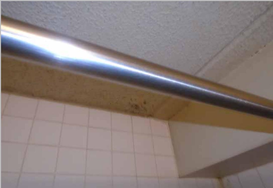
Remove Mildew in Unit 804 Bathroom Ceiling (Non-Critical Repair)
