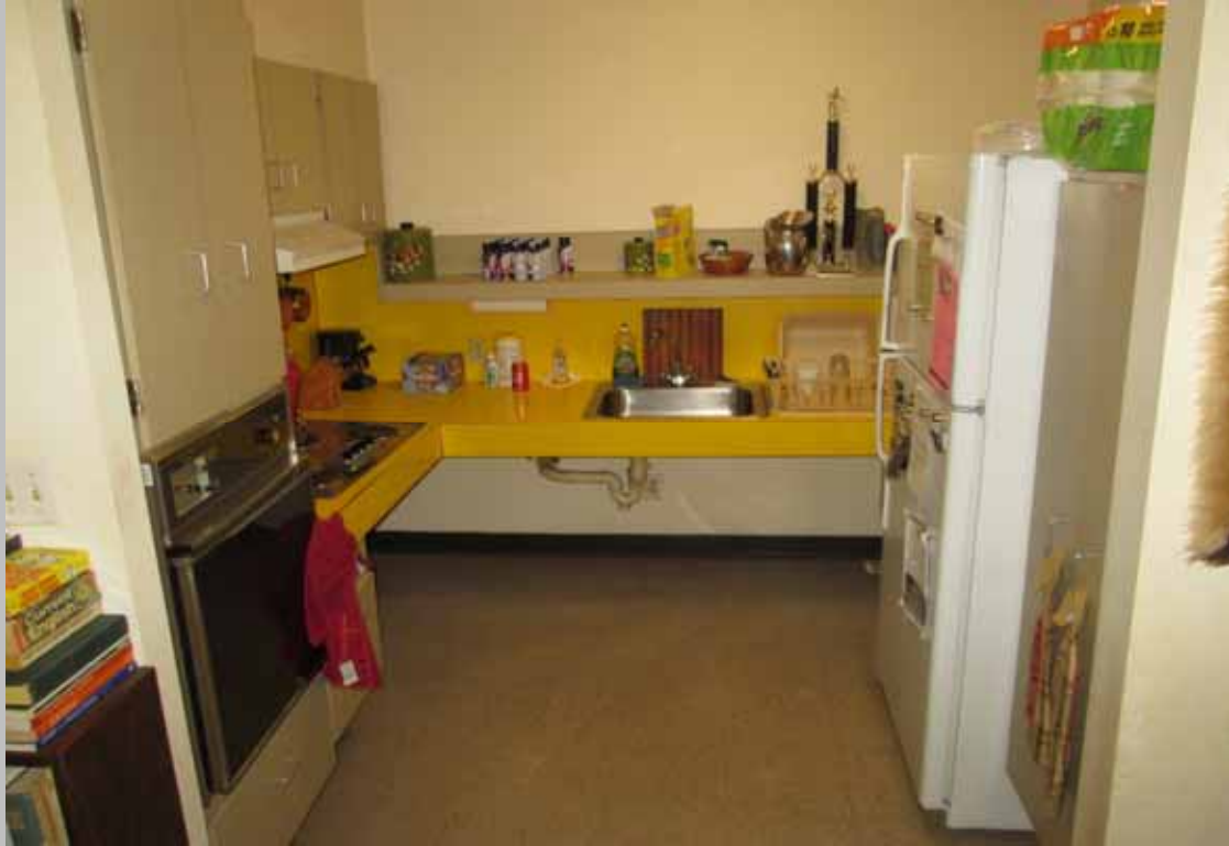
View of the kitchen within designated handicapped dwelling unit 102 – featuring compliant clear floor space and roll-under access to the sink and electric cook-top
