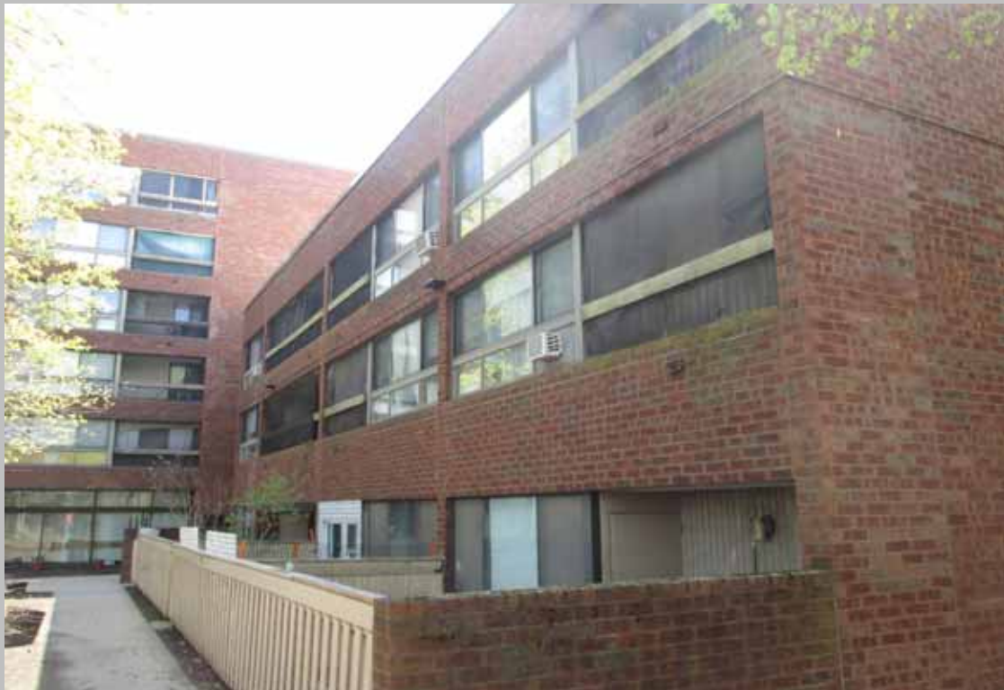
View of a portion of mildew growth on the building exterior in need of pressure washing (Non-Critical Repair)
