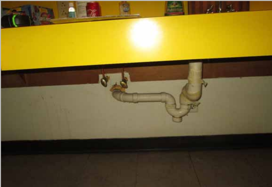
View of a typical HC dwelling unit kitchen sink without scald and abrasion protection on piping (Critical Repair)
