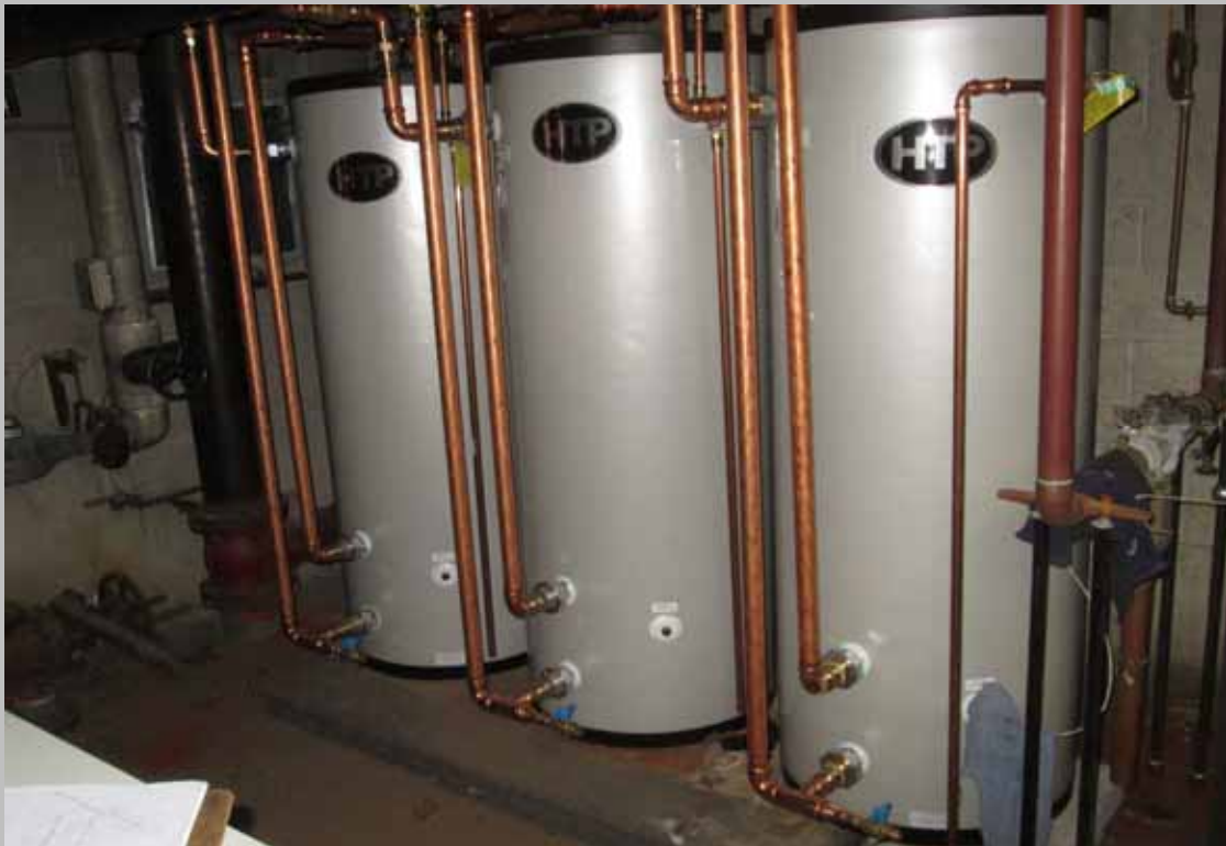
View of DHW storage tanks
