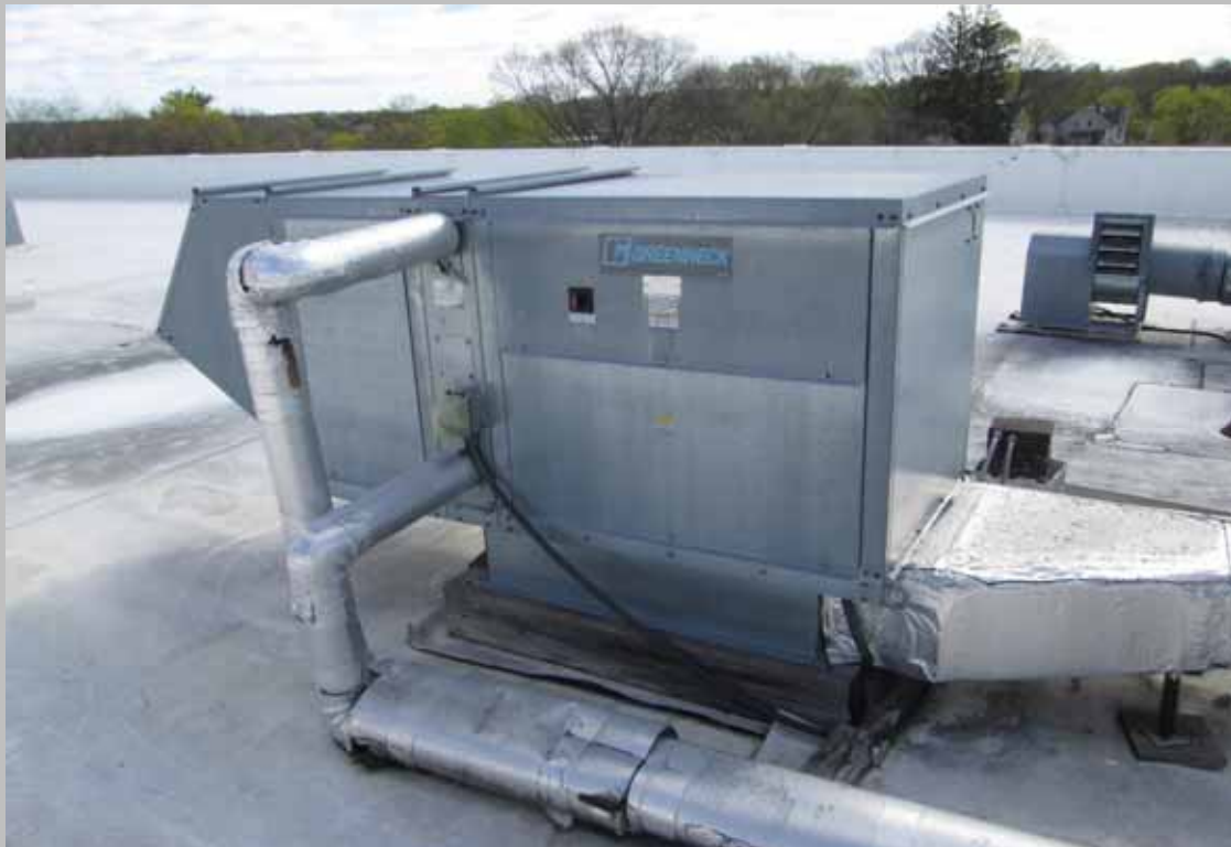
View of roof mounted make-up unit
