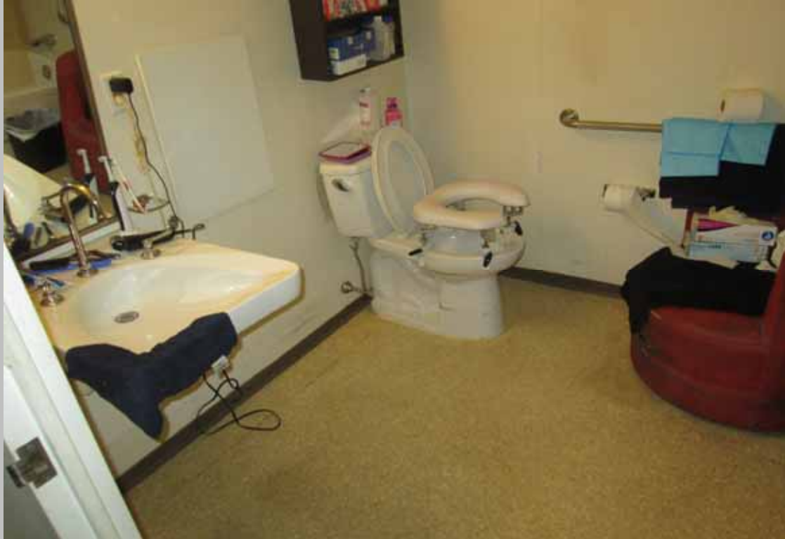
View of the bathroom within designated handicapped dwelling unit 102 – featuring compliant clear space and a roll-under sink with levered handle hardware
