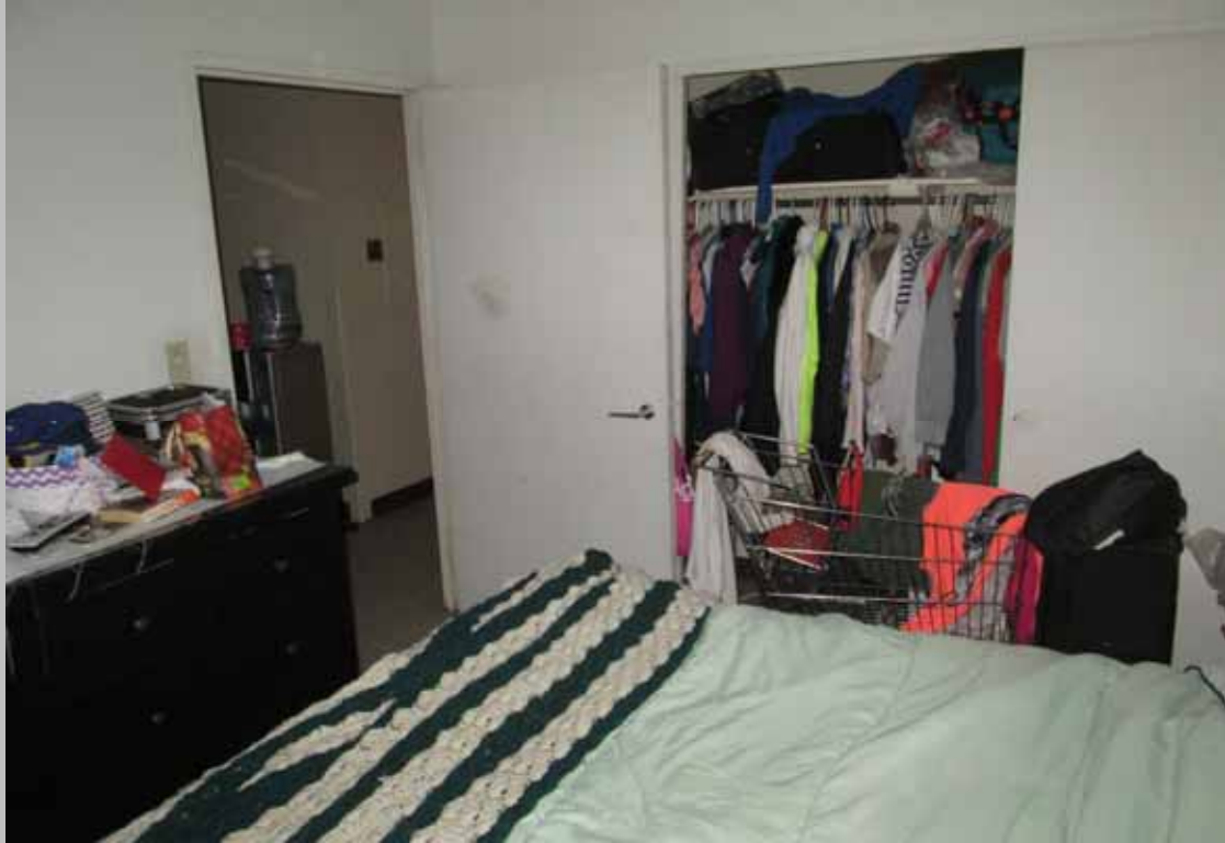
View of the bedroom within designated handicapped dwelling unit 201 – featuring 18-inches at the pull side of the entry door and levered handle hardware
