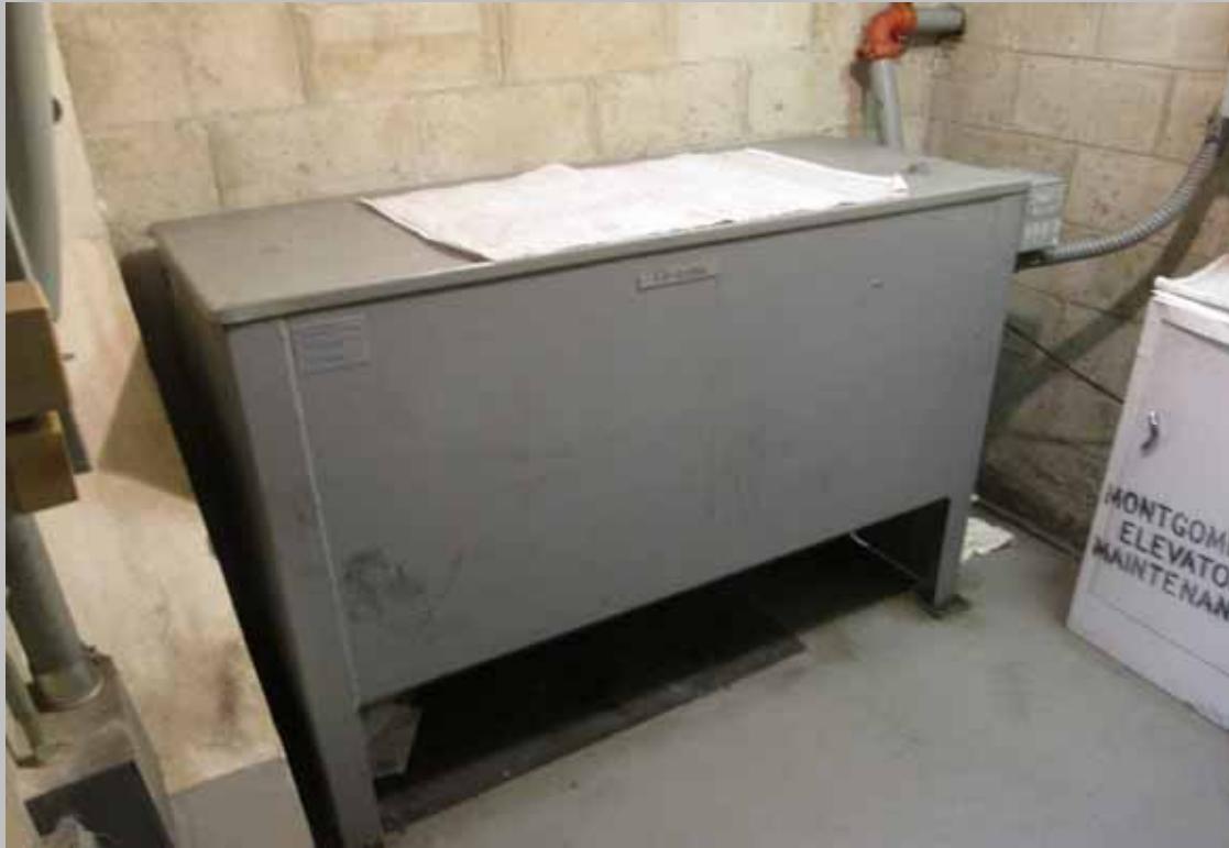
View of elevator equipment
