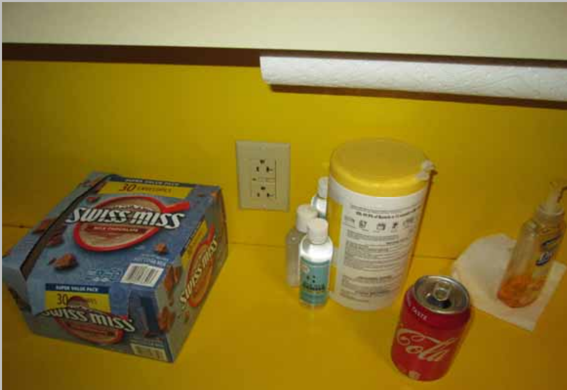
View of GFCI electrical outlet – dwelling unit
