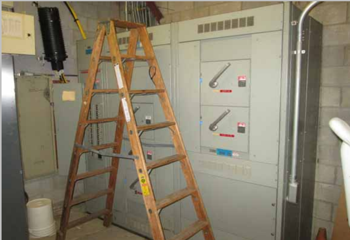
View of electrical switchgear
