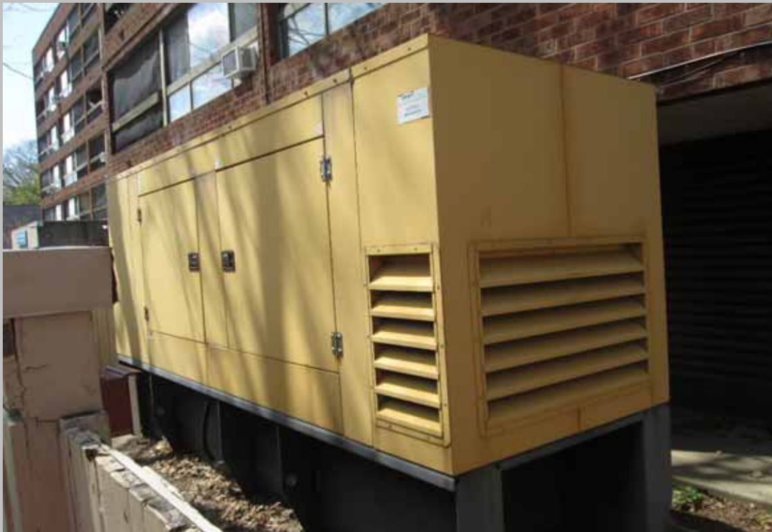
View of the building emergency generator
