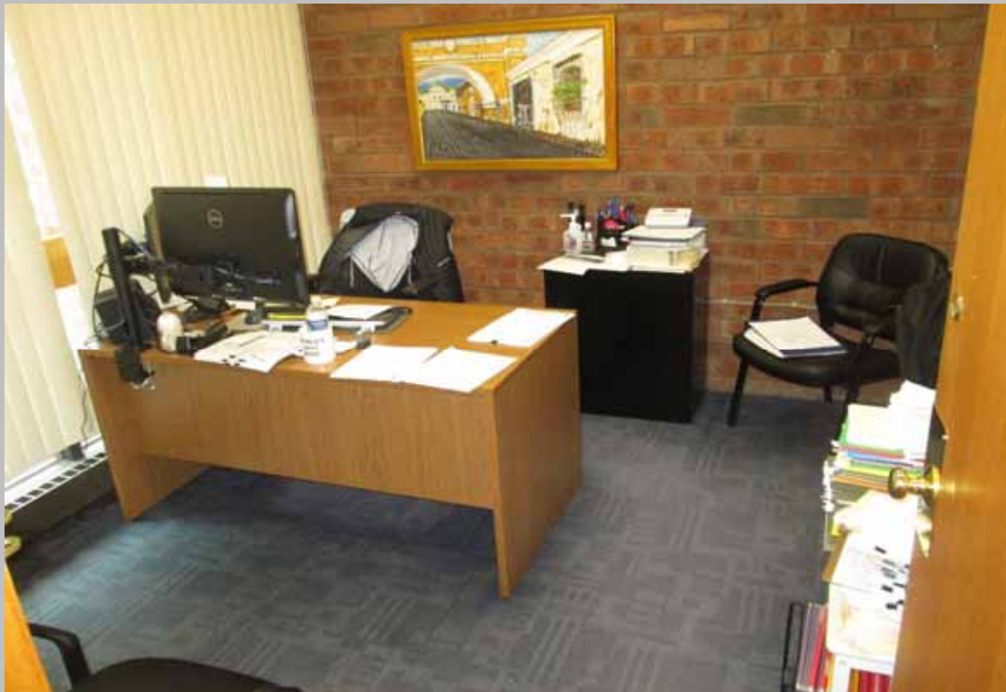
View of the property manager's office – featuring non-compliant knobbed entry door hardware (Critical Repair)
