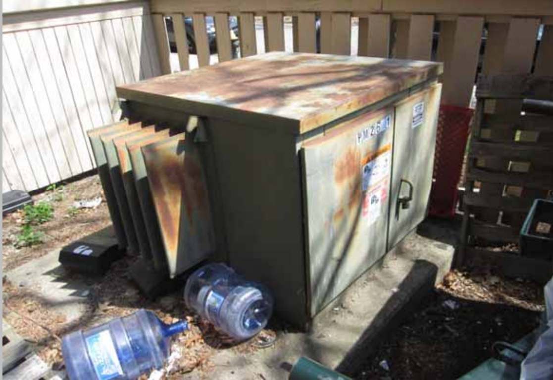
View of pad mounted electrical transformer
