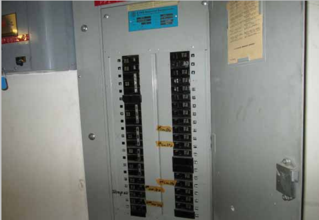
View of an electric breaker panel
