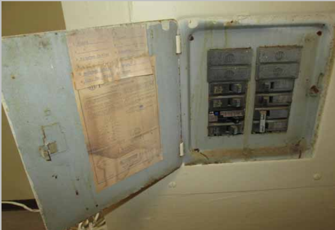
View of electric breaker panel - dwelling unit
