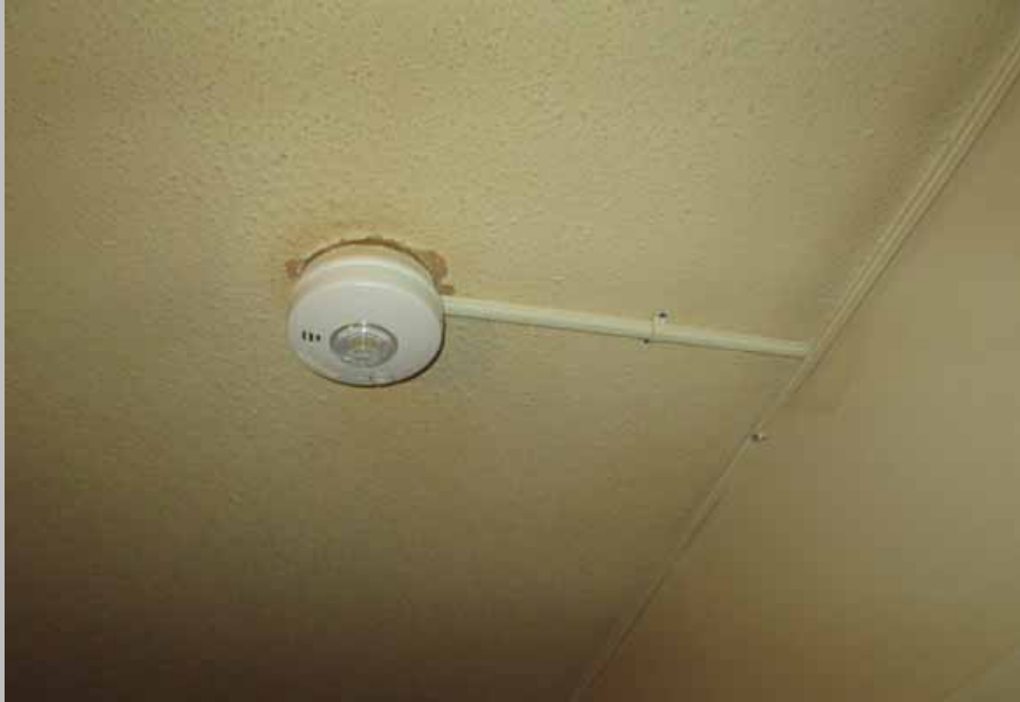
View of smoke detector – dwelling unit
