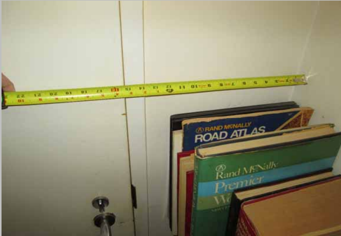
View of 16-inches at the pull-side of the primary entry door at HC Unit 102 (Critical Repair)
