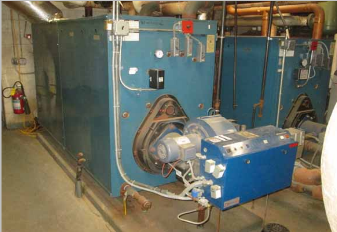
View of the heating boilers
