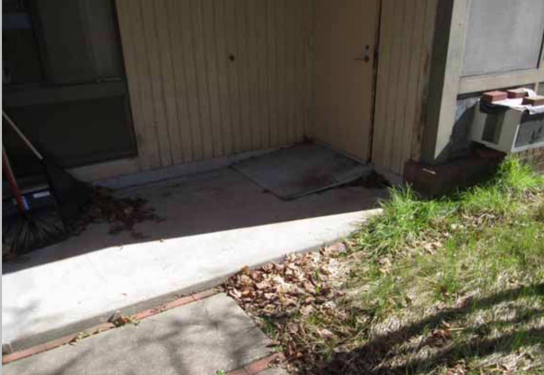
View of the non-compliant patio ramp at HC unit 102
