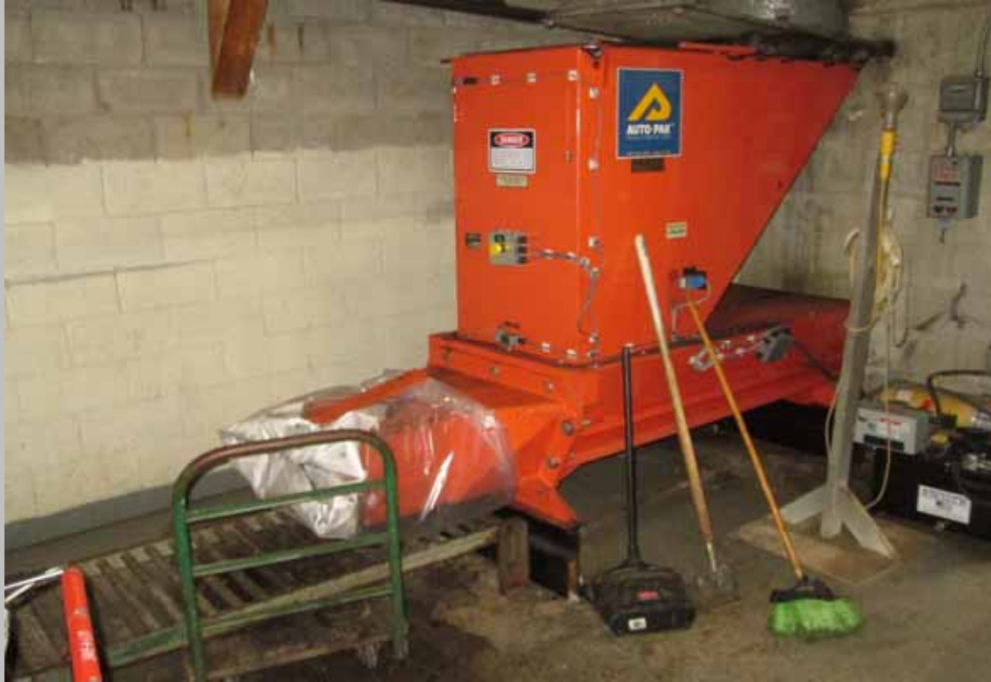
View of the trash compactor
