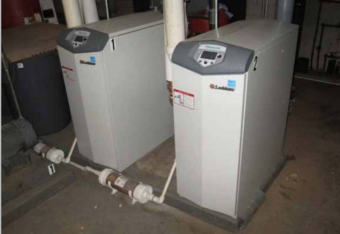
View of high efficiency DHW boilers
