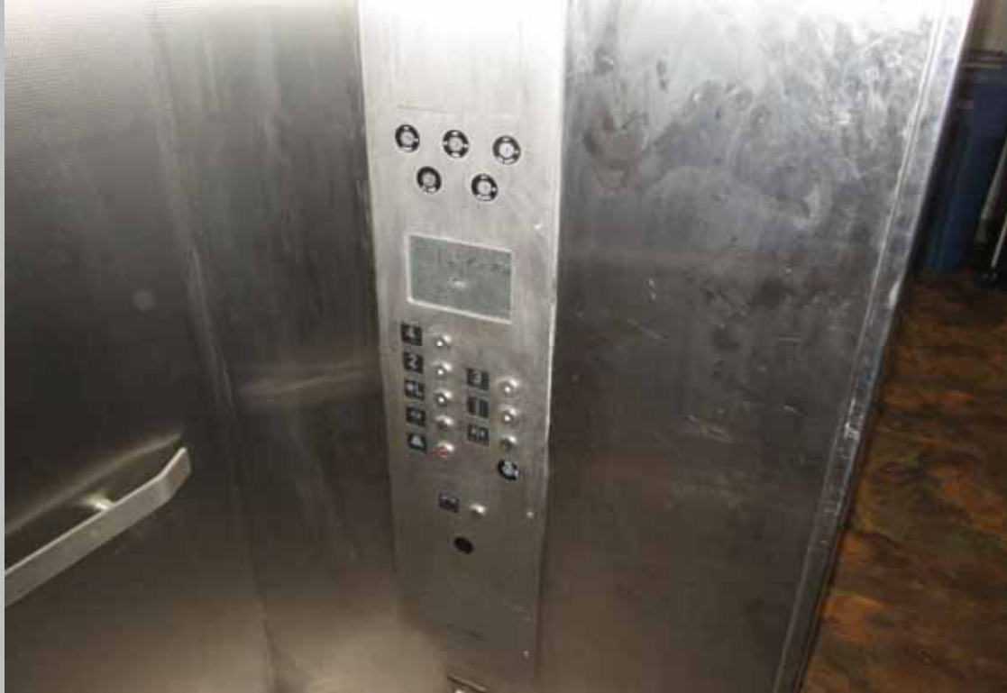
View of an elevator cab
