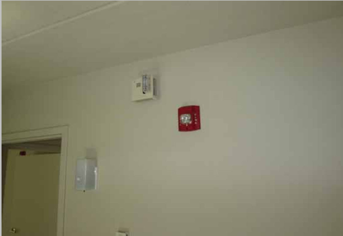
View of an A/V alarms - dwelling unit
