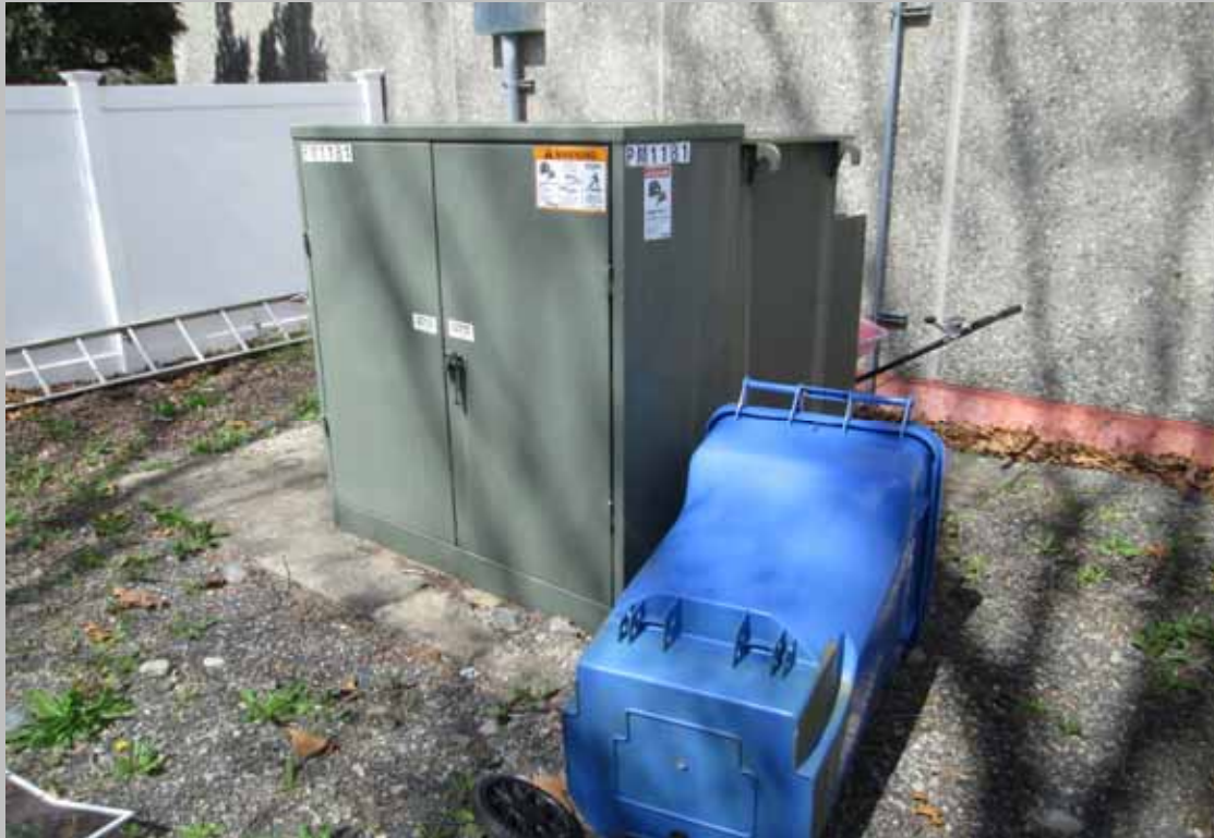
View of pad mounted electrical transformer
