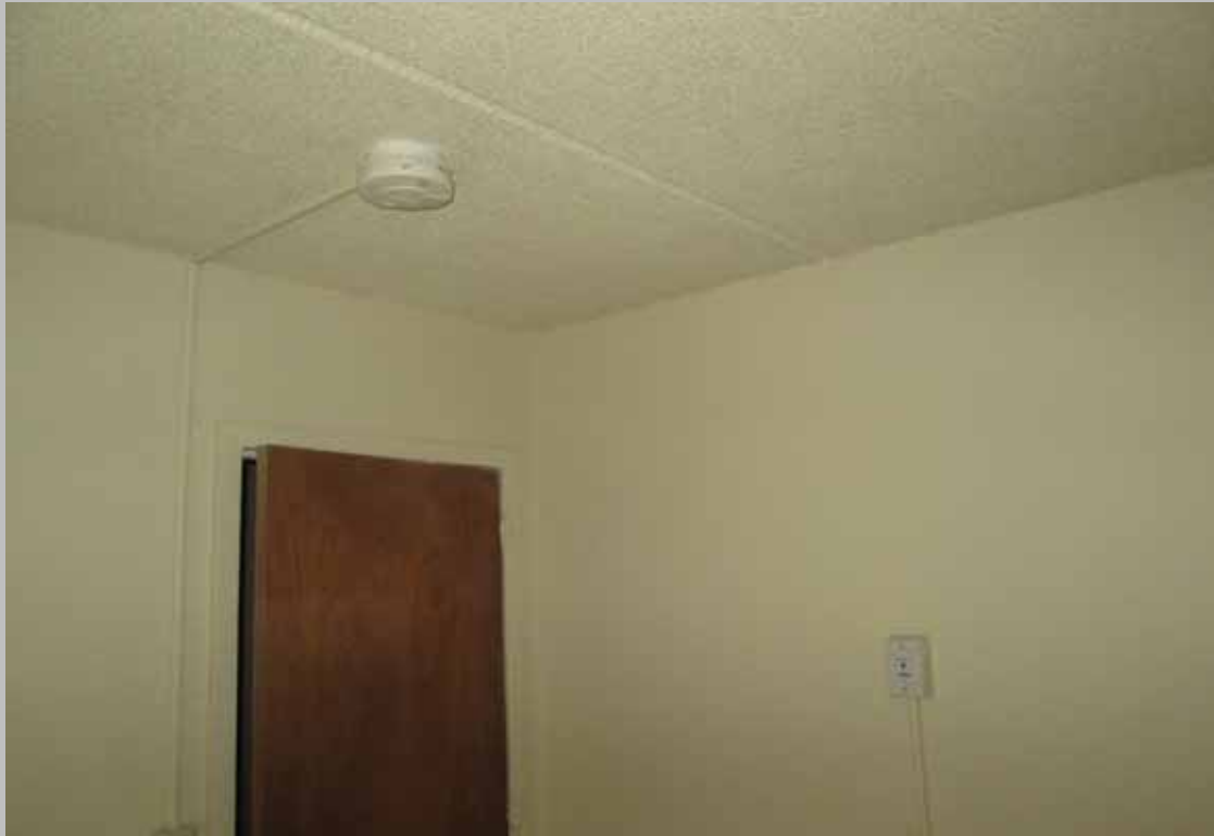
View of a smoke detector - dwelling unit
