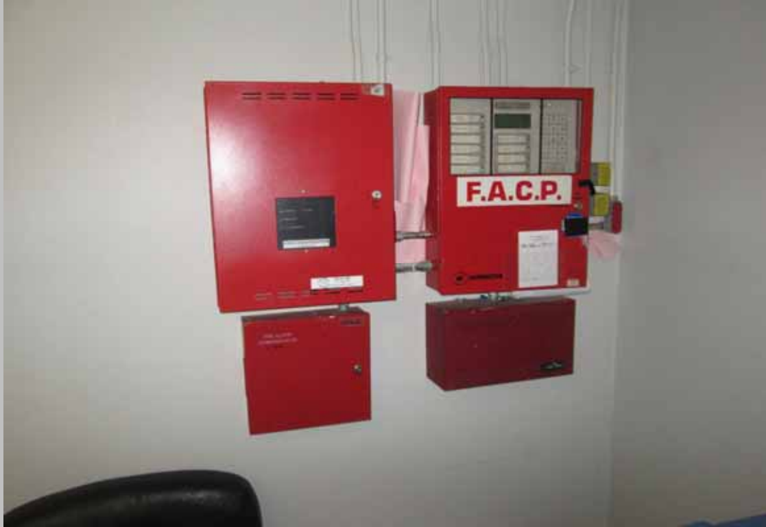
View of fire alarm control panel
