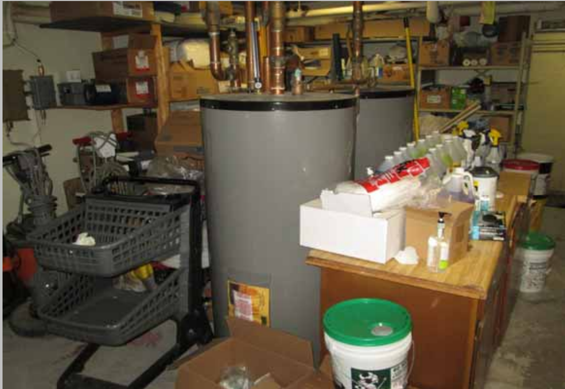
View of water storage tanks
