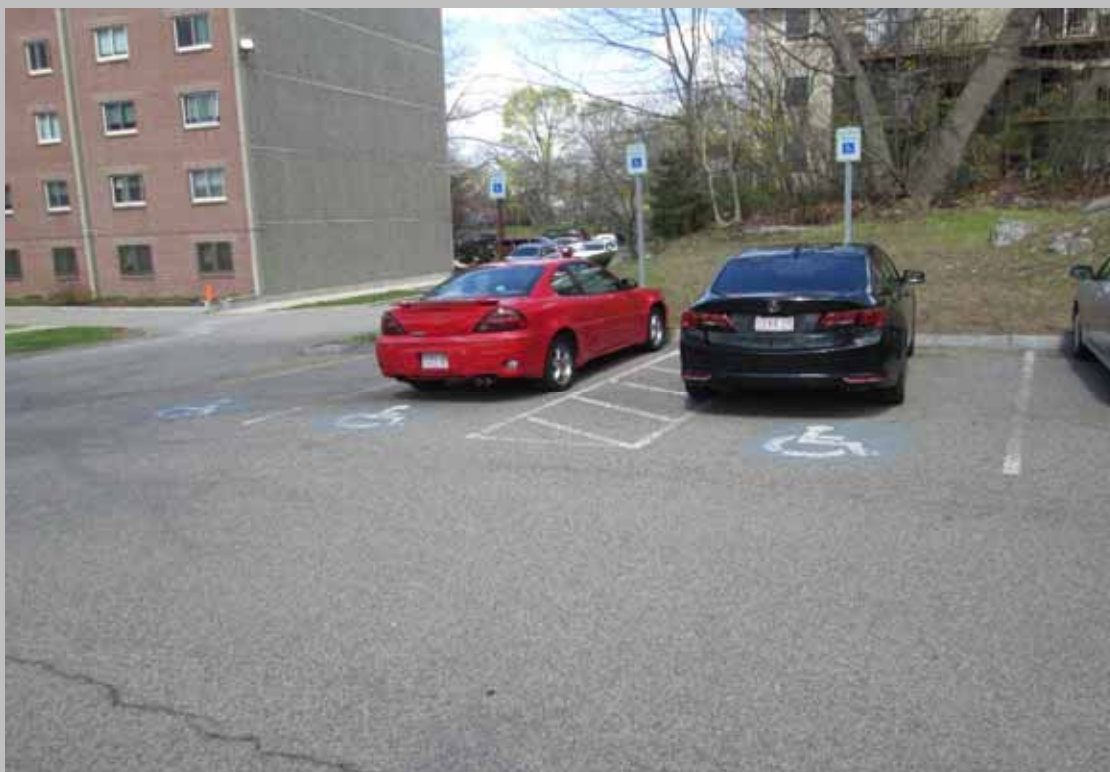
View of existing handicapped parking lacking a van accessible space (Critical Repair)
