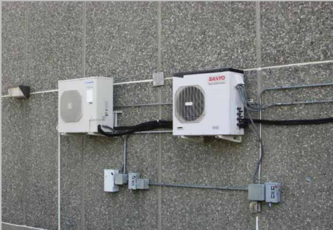
View of mini-split HVAC units
