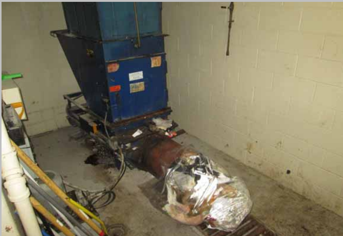
View of the trash compactor
