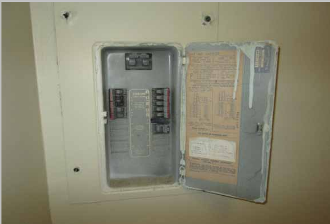
View of an electric breaker panel - dwelling unit
