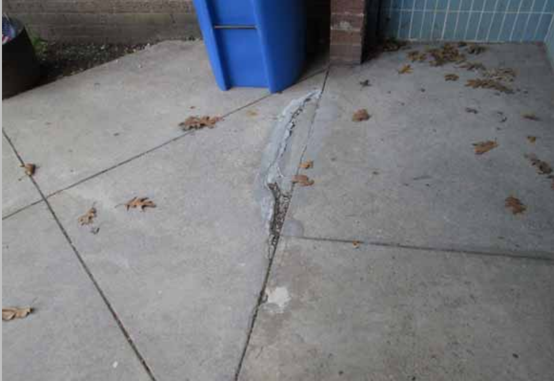
View of the trip hazard located outside of the main entry door (Critical Repairs)
