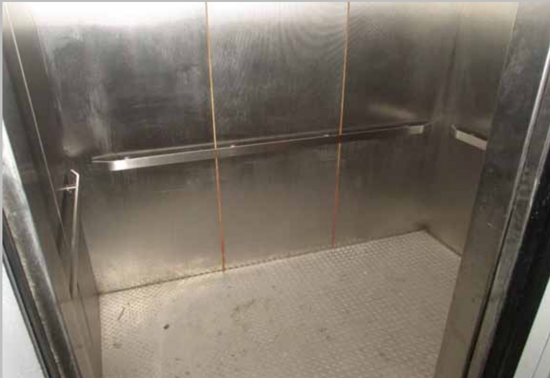
View of an elevator cab
