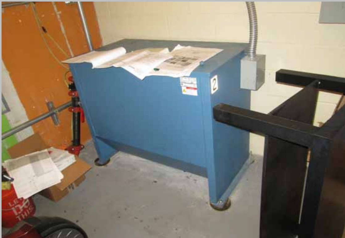
View of the elevator equipment
