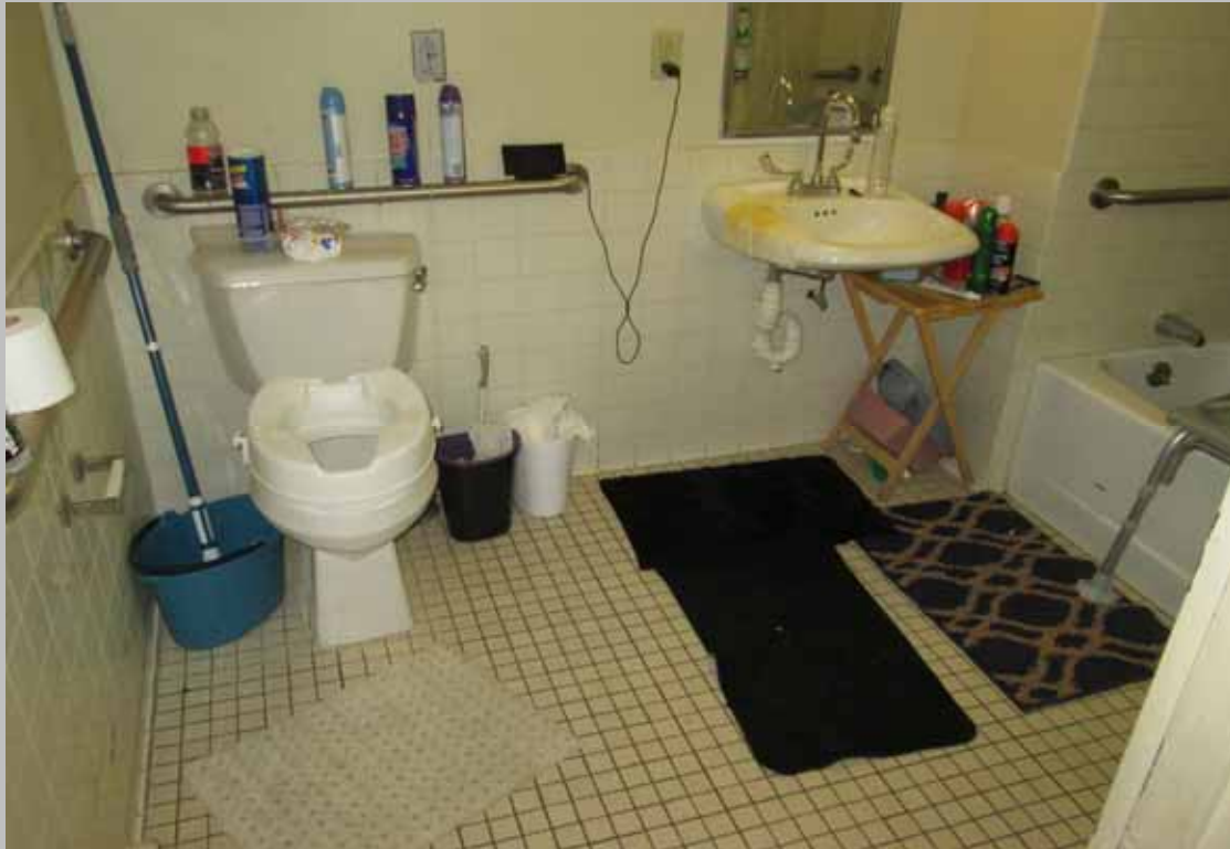
View of the bathroom within designated handicapped Unit 35 featuring compliant side and rear grab bars at the toilet and compliant clear floor space
