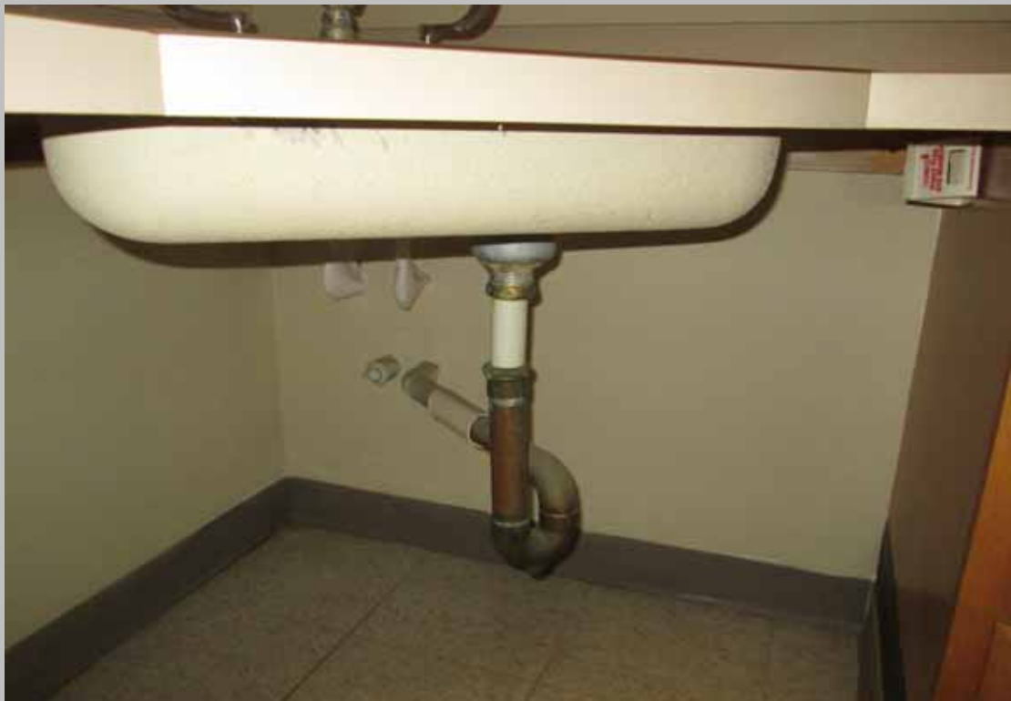
View of kitchen sink in HC Unit 17 without scald and abrasion protection (Critical Repair)
