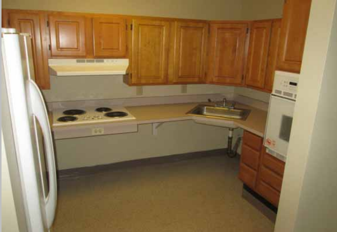
View of the kitchen within designated handicapped dwelling unit 17 featuring roll-under sink and cook-top, levered handle sink hardware, and compliant clear floor space
