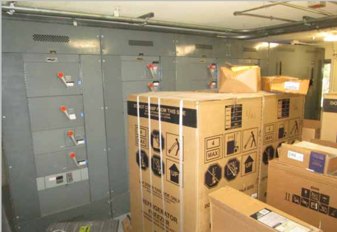
View of switchboard
