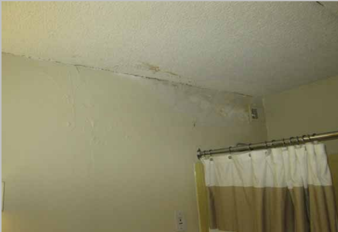
View of water damage in Unit 43 (Non-Critical Repair)
