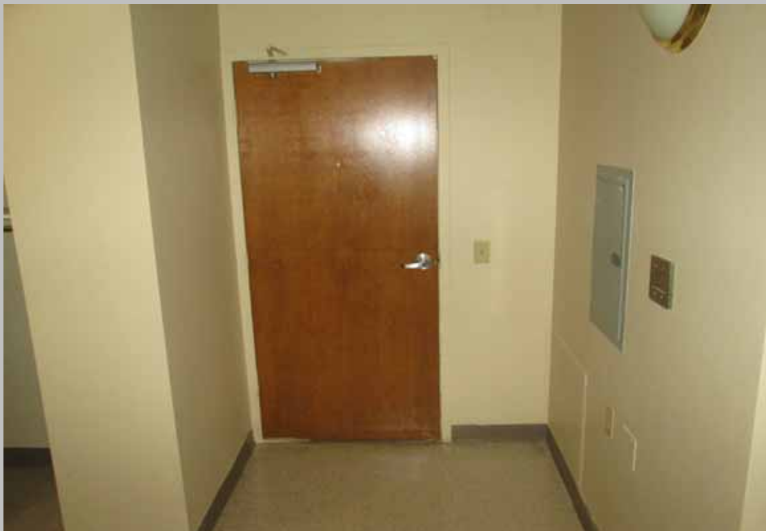
View of the entrance area within designated handicapped dwelling unit 17 featuring compliant levered door hardware and 18-inches at the pull-side of the door
