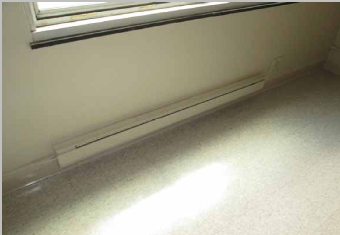
View of electric baseboard heater - dwelling unit
