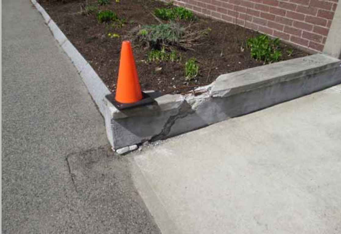
View of damaged concrete wall at south sidewalk (Non-Critical Repairs)
