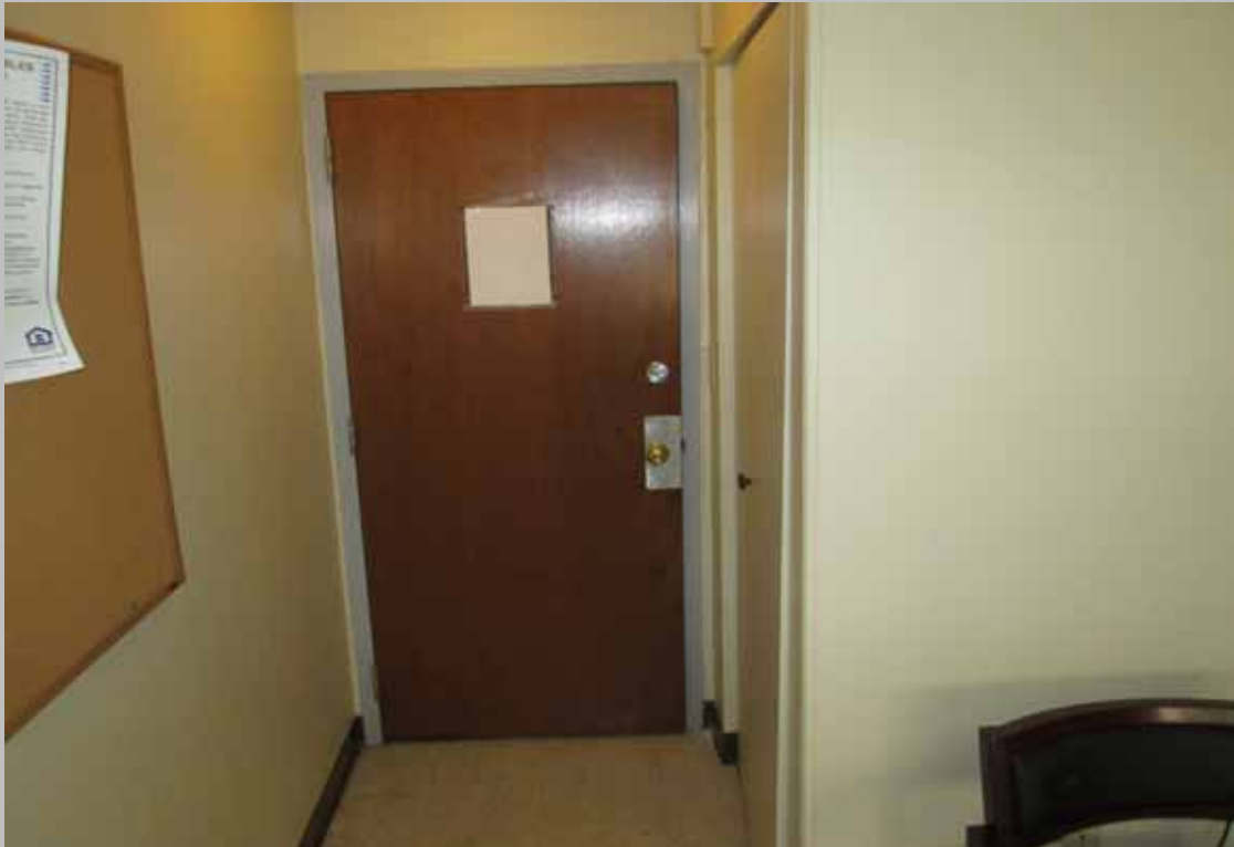
View of management office door without 18-inches clear maneuvering space and lacking levered hardware (Critical Repairs)
