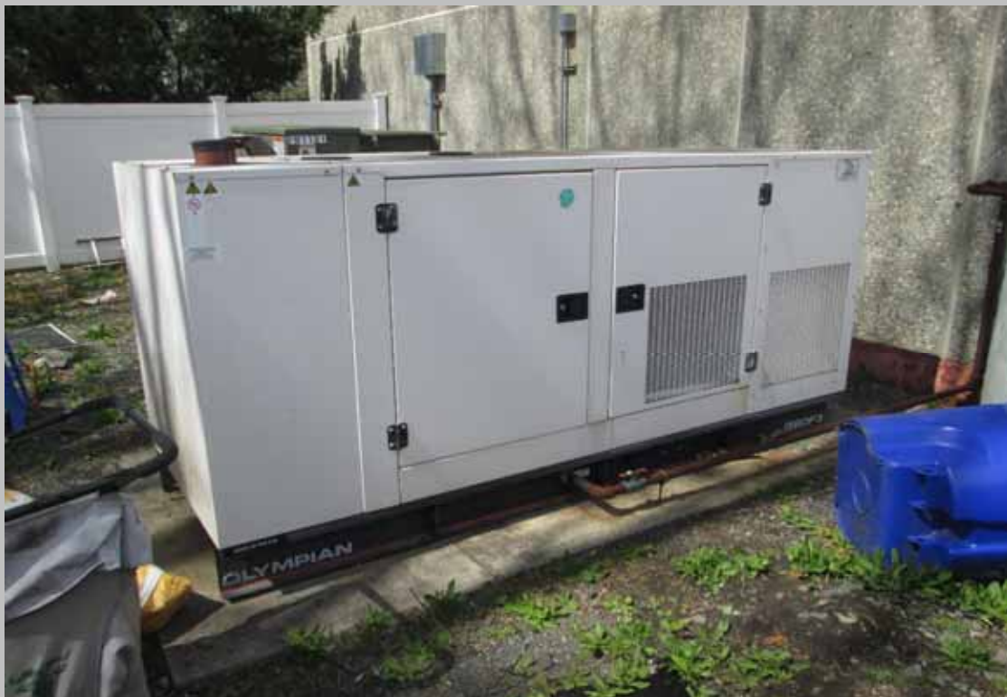
View of the emergency generator
