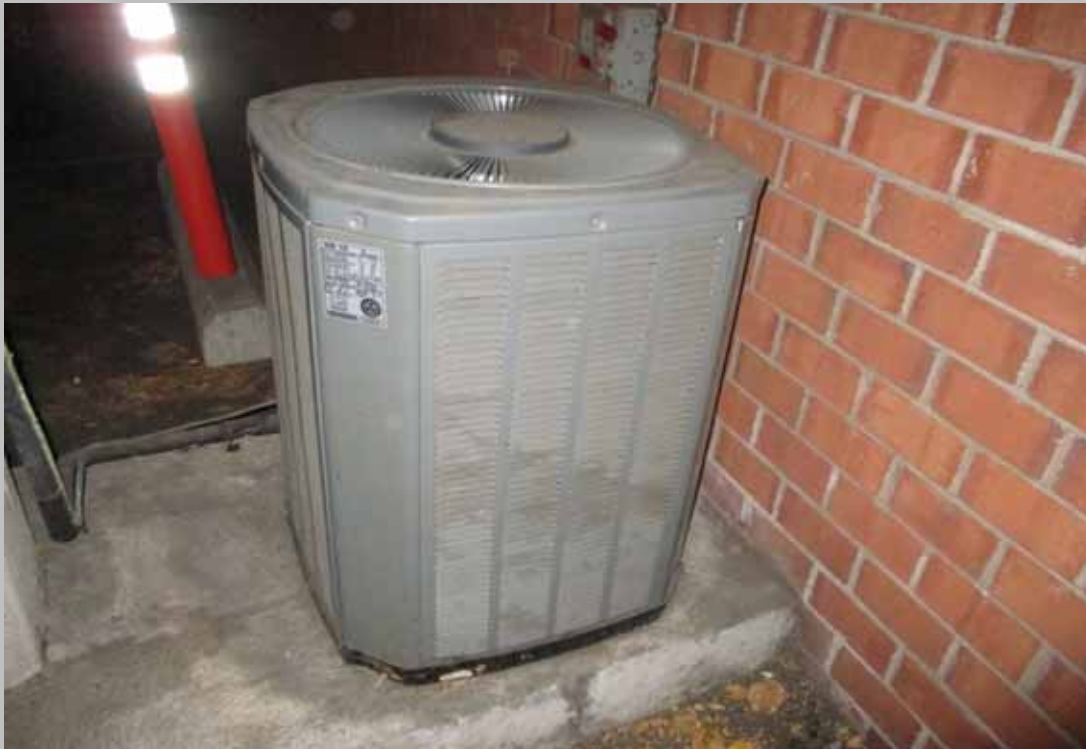
One of three ground-mounted condensers.
