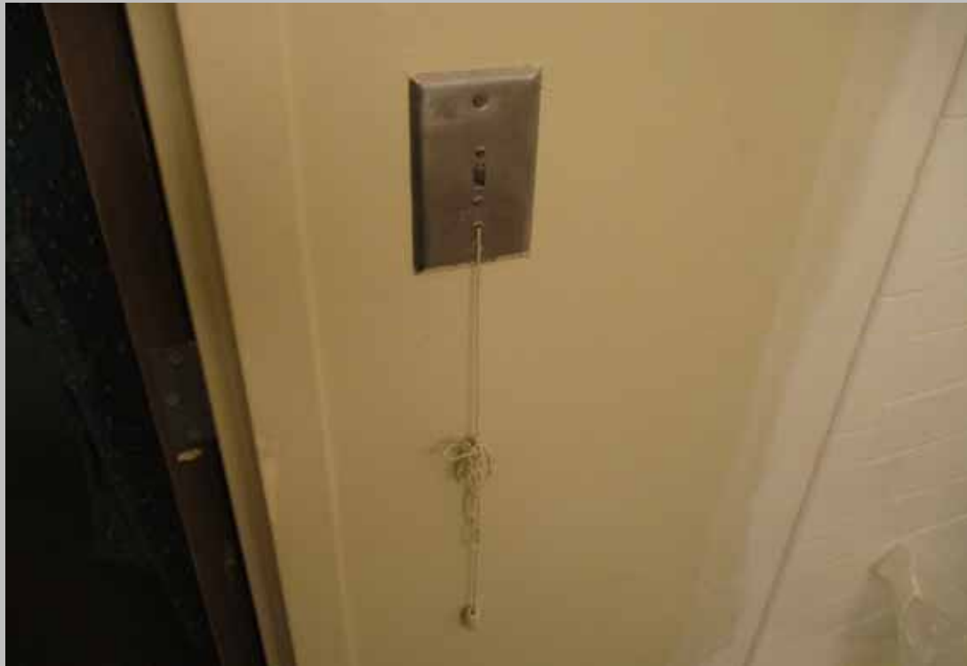
Example of emergency call pull-cord system in bathrooms.
