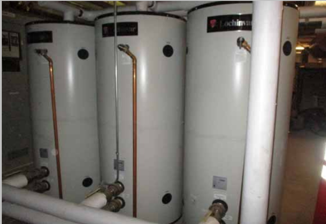
Three hot water holding tanks.
