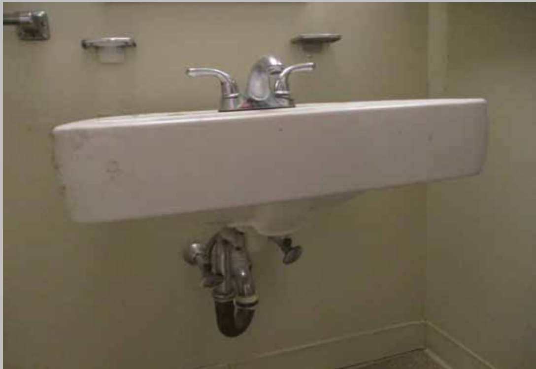
Bathroom sink missing scald proof piping.
