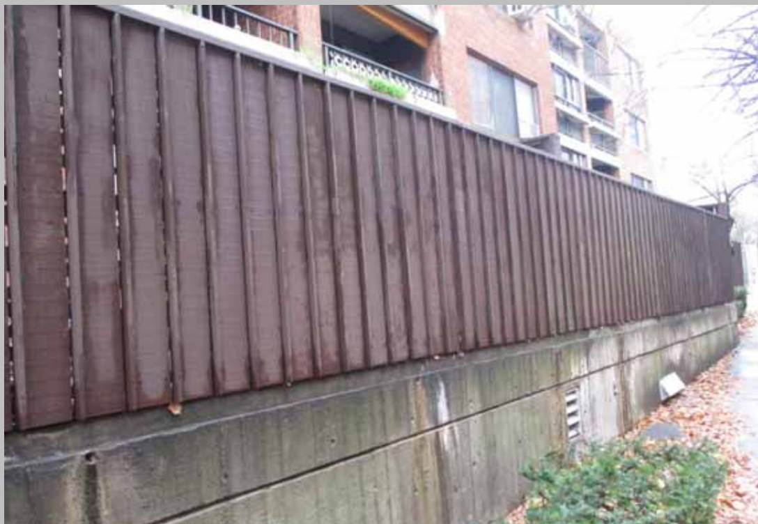
Concrete wall and wood privacy fence along northern, eastern, and southeast side of building.
