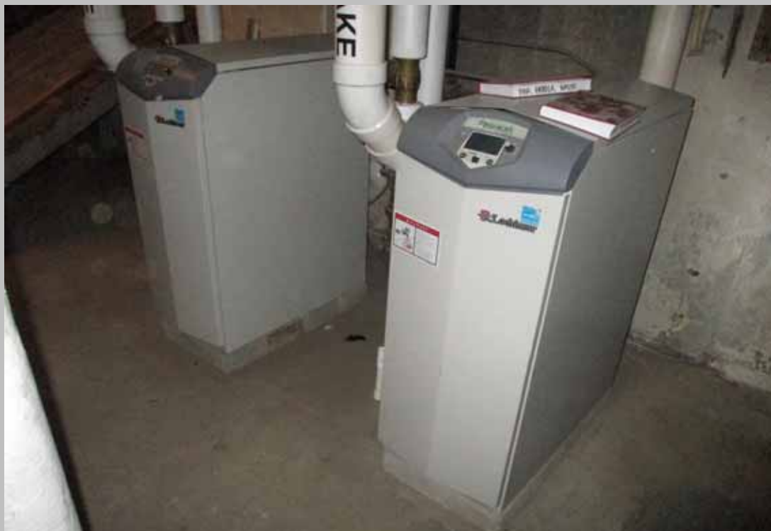
Boilers for domestic hot water.
