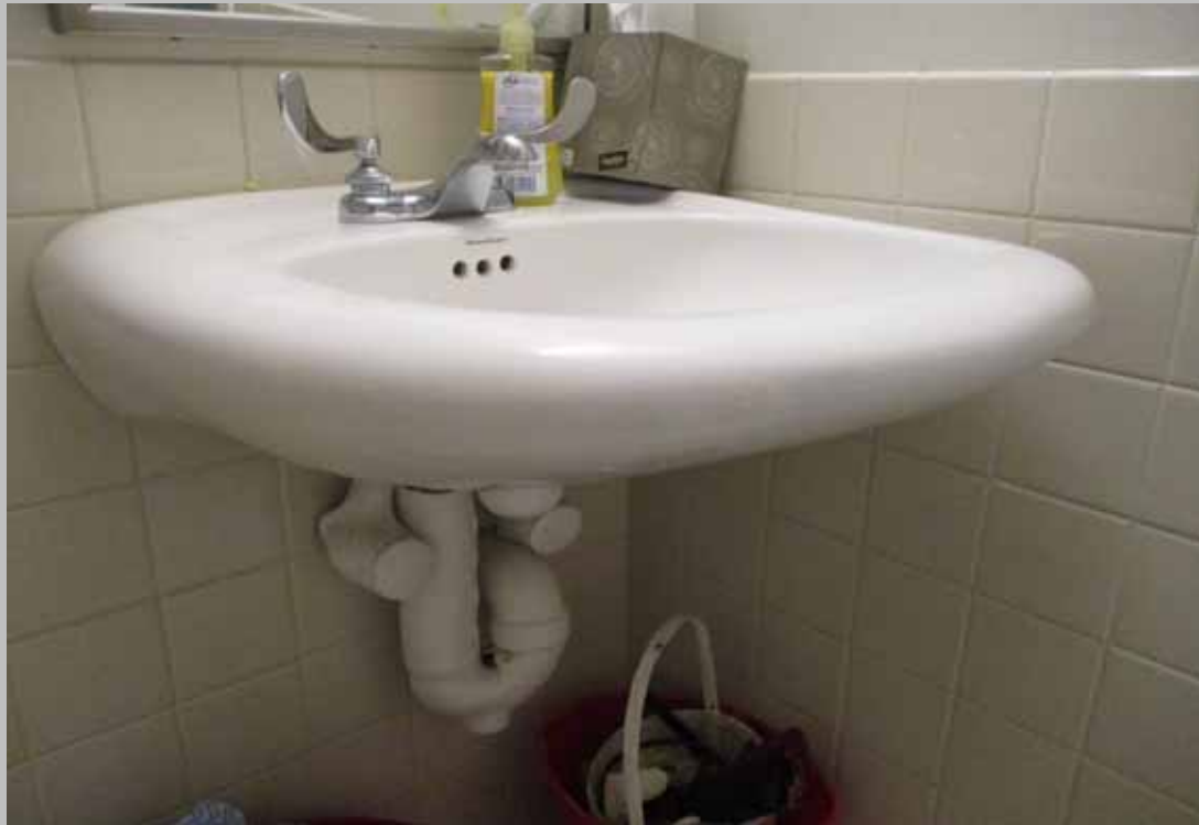
Correct scald proof piping in bathroom Unit 227
