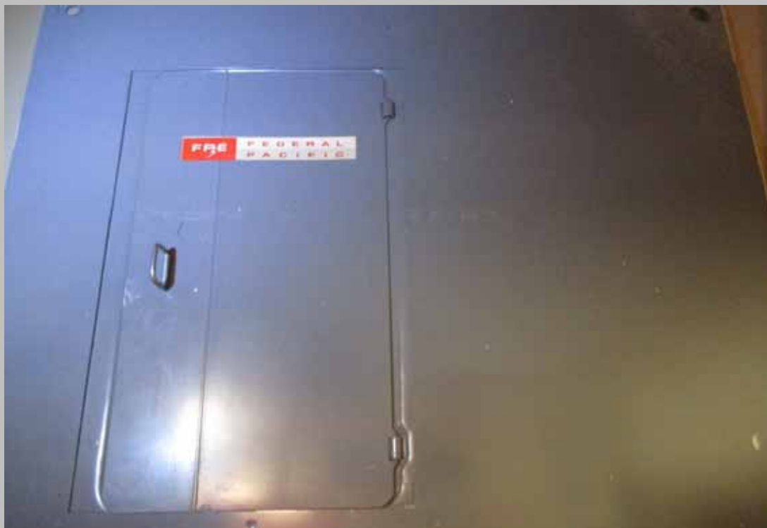
Example of Federal Pacific circuit breaker panel.
