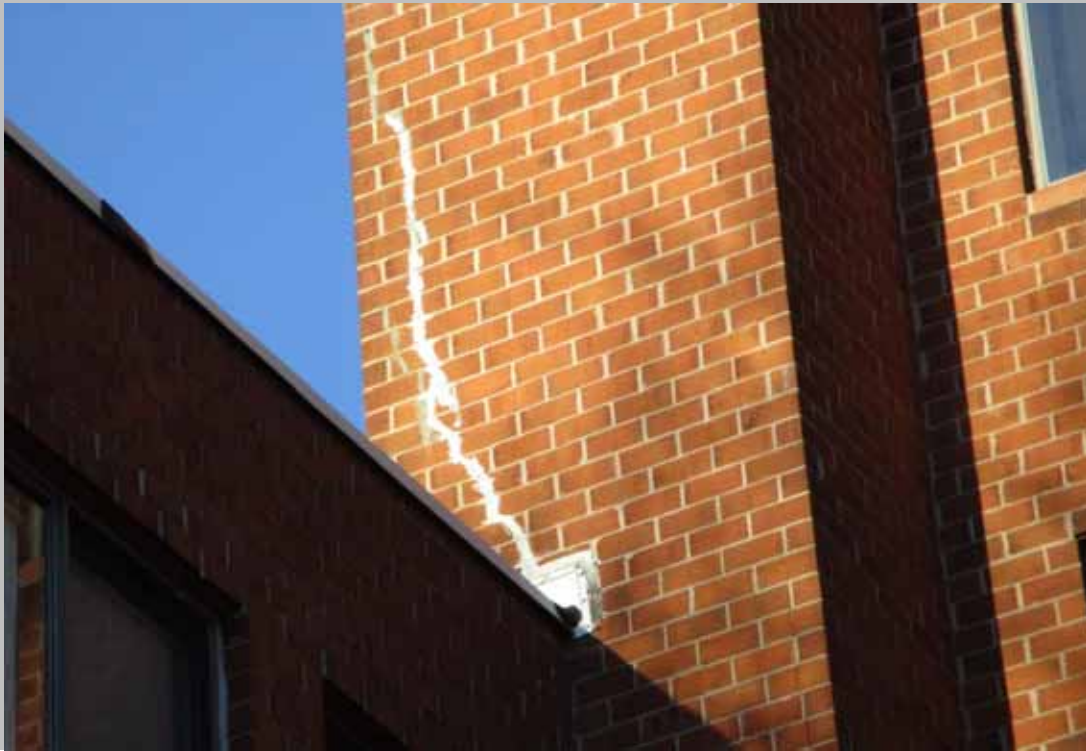
Evidence of another crack repair in upper brick work.
