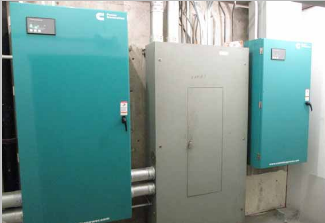
Generator control panels.
