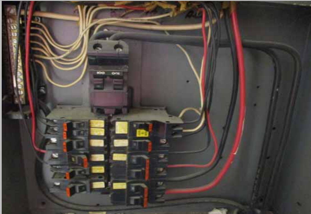
Inside of a typical Federal Pacific circuit breaker panel.
