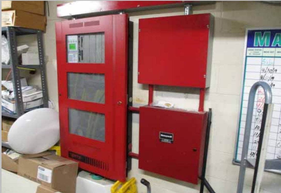
Main fire panel.
