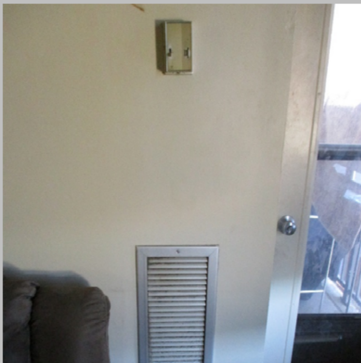
Fan coil unit in apartment.
