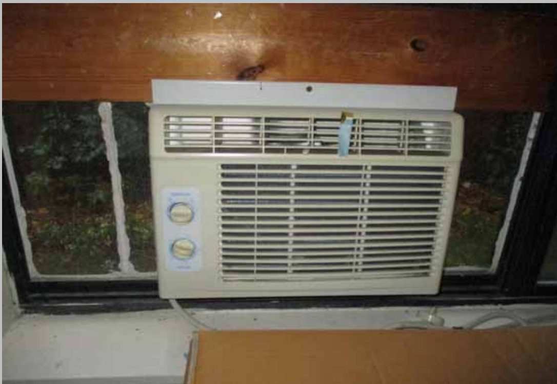
Typical window-mounted A/C unit in apartments.
