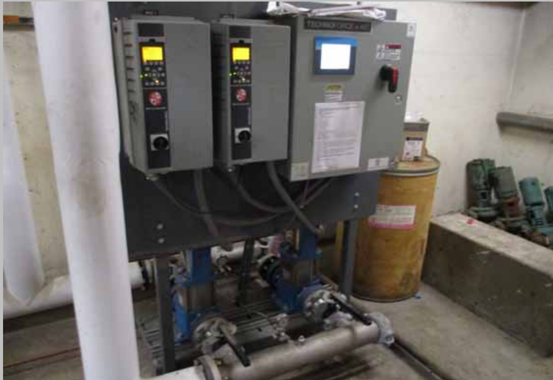
Domestic water circulating system.
