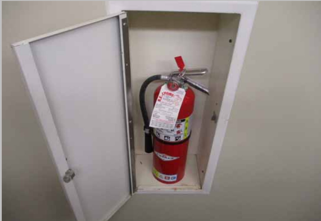
Typical fire extinguisher throughout building.
