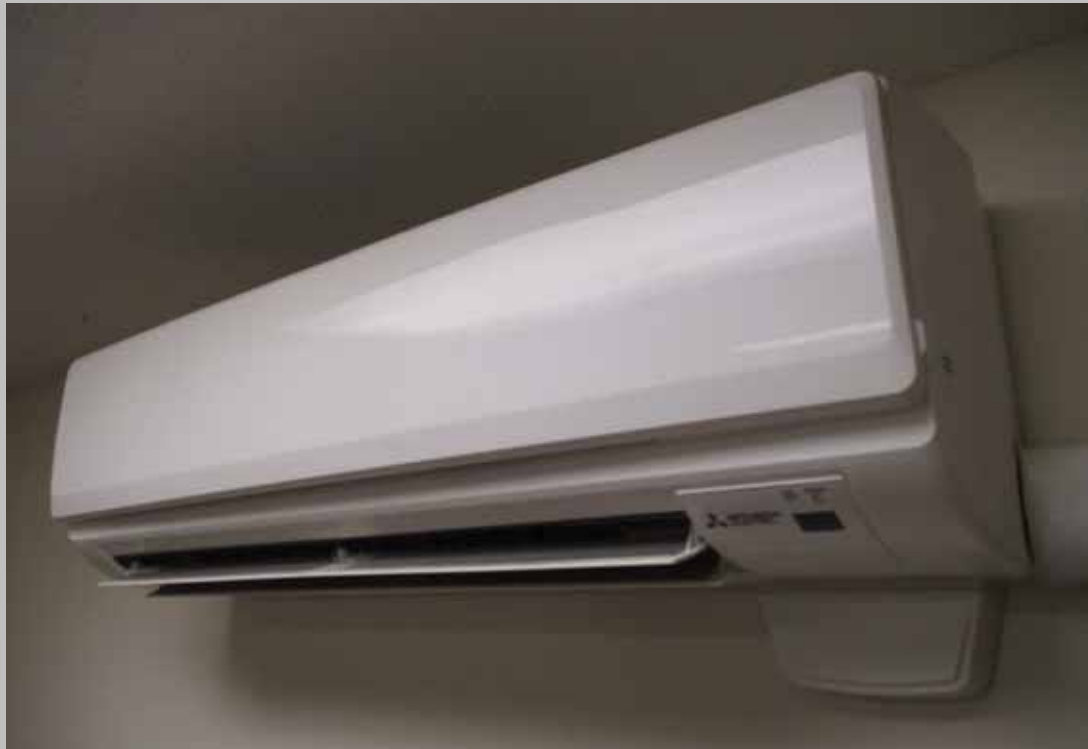
Ductless units in Task Force offices.
