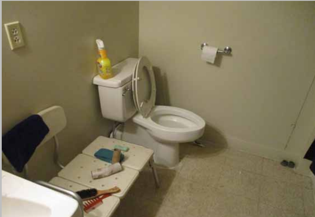
Toilet missing grab bars Unit 221.
