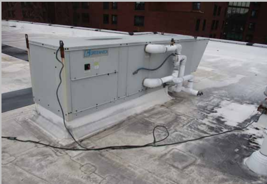
One of the Greenheck make-up air systems.
