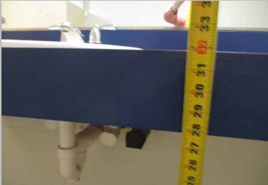
Correct sink height, levered hardware, and scald proof piping.
