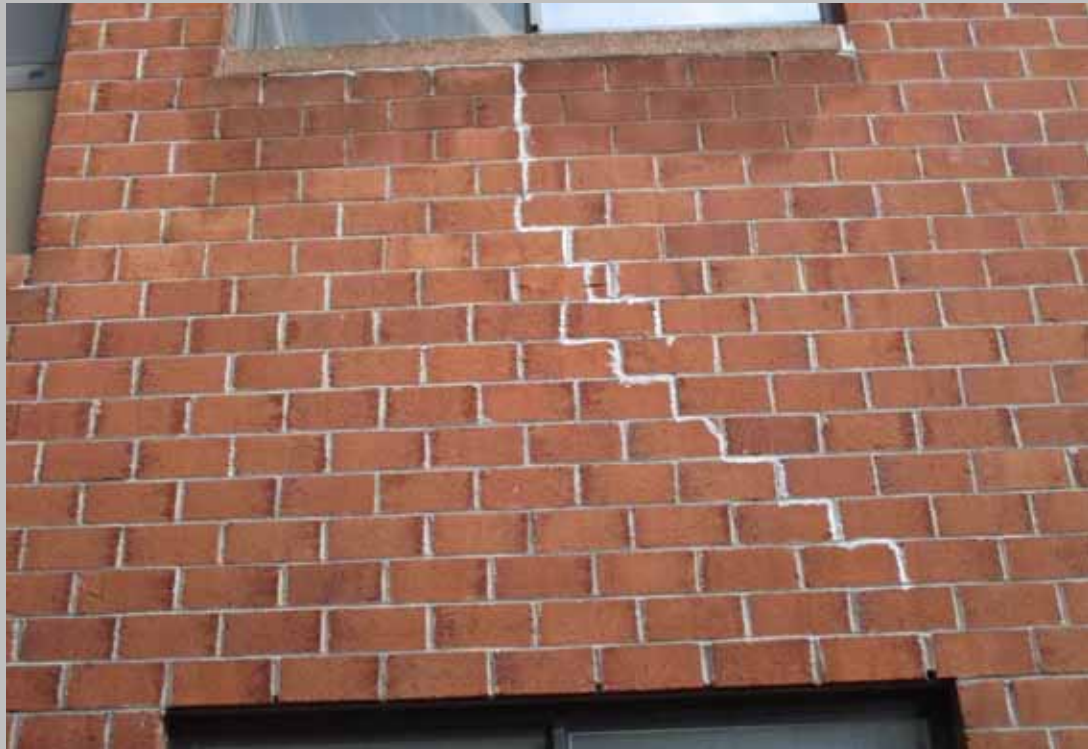
Step crack in brick façade, inner southeastern side of building by carport entrance.
