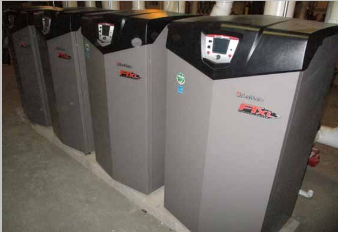
Hot water boilers for heating.
