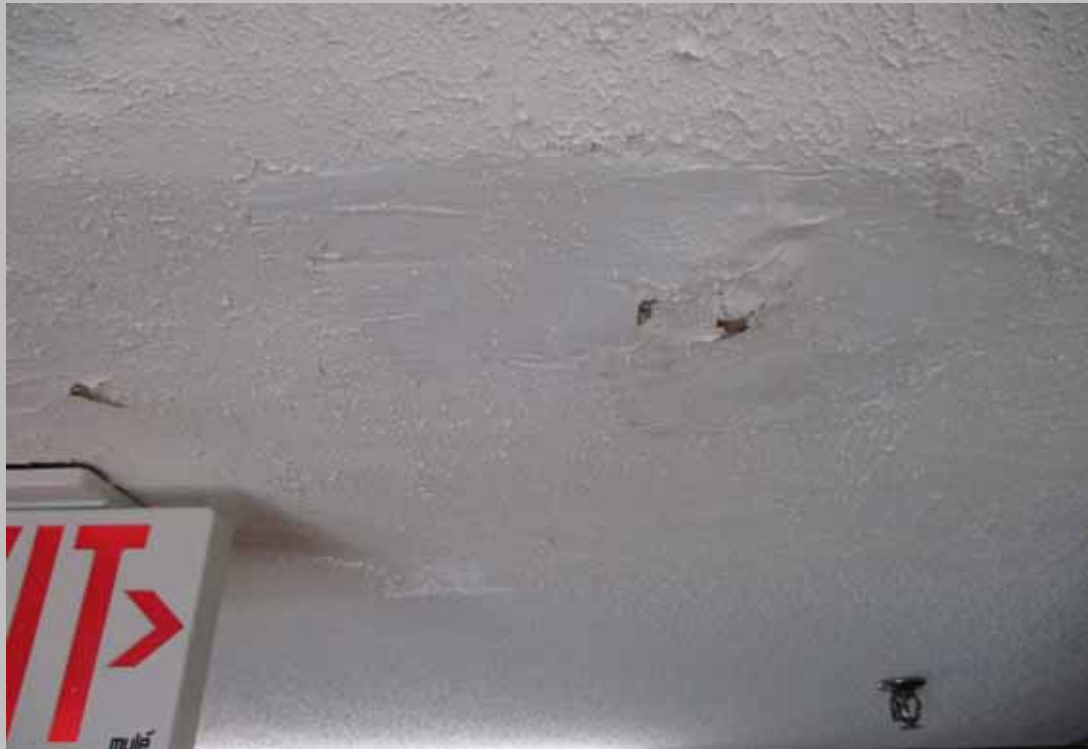
Another view of ceiling water penetration 5 th floor corridor.
