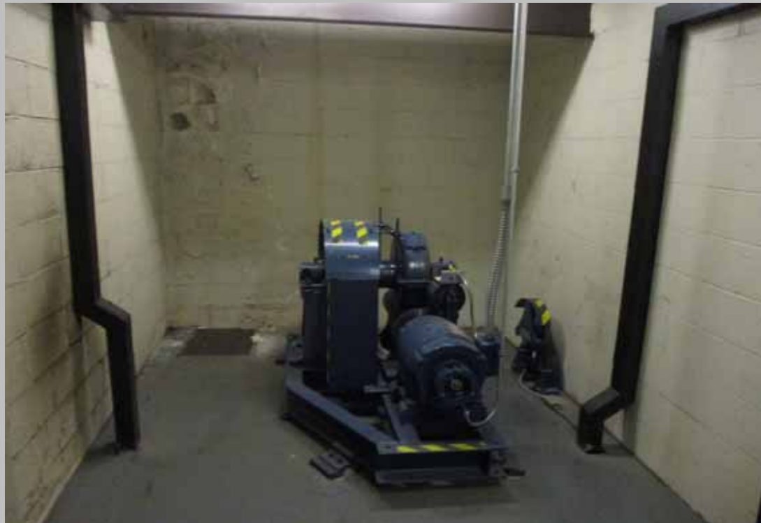
Overhead traction elevator machinery.
