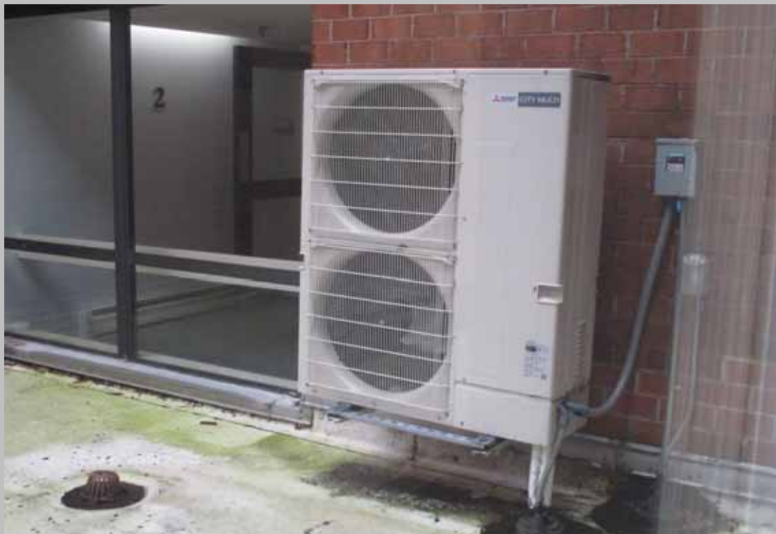
Condensers for ductless units.
