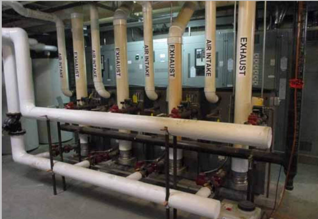
Back side of heating hot water boilers.
