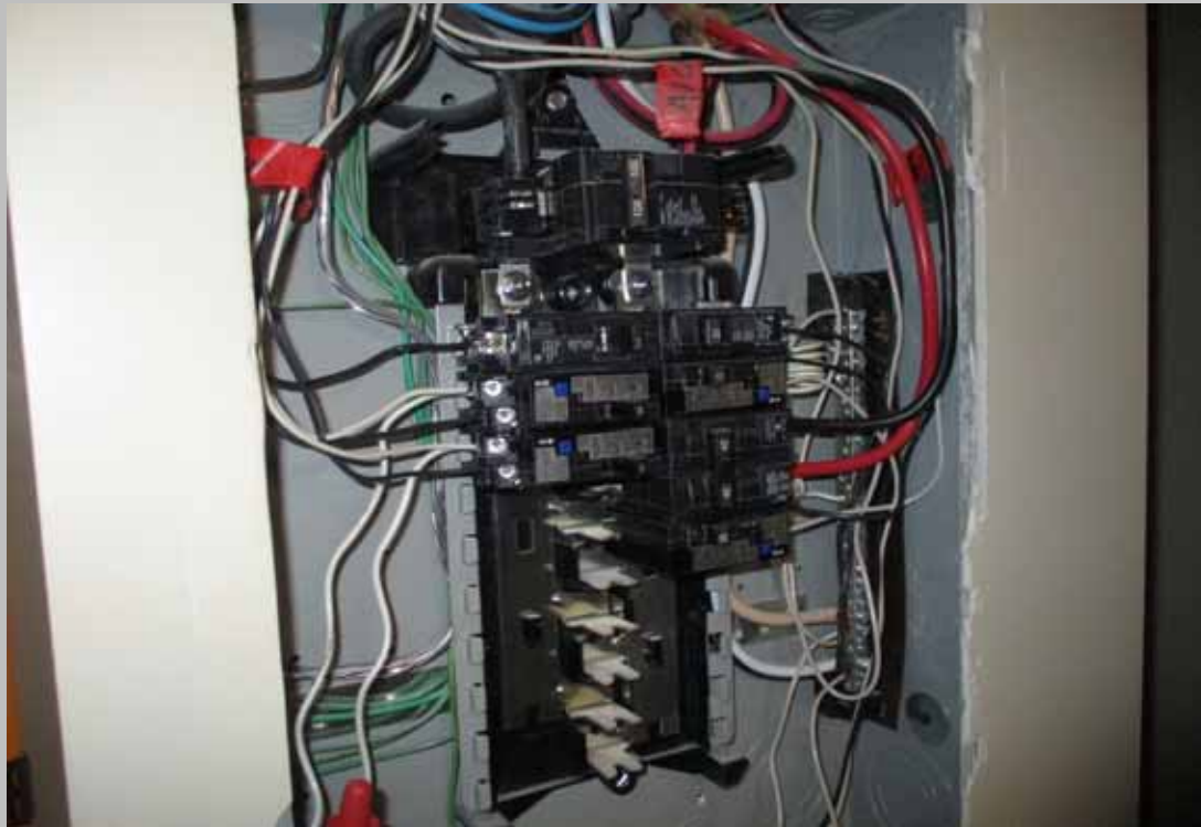
Example of newer circuit breaker panel in select apartments.
