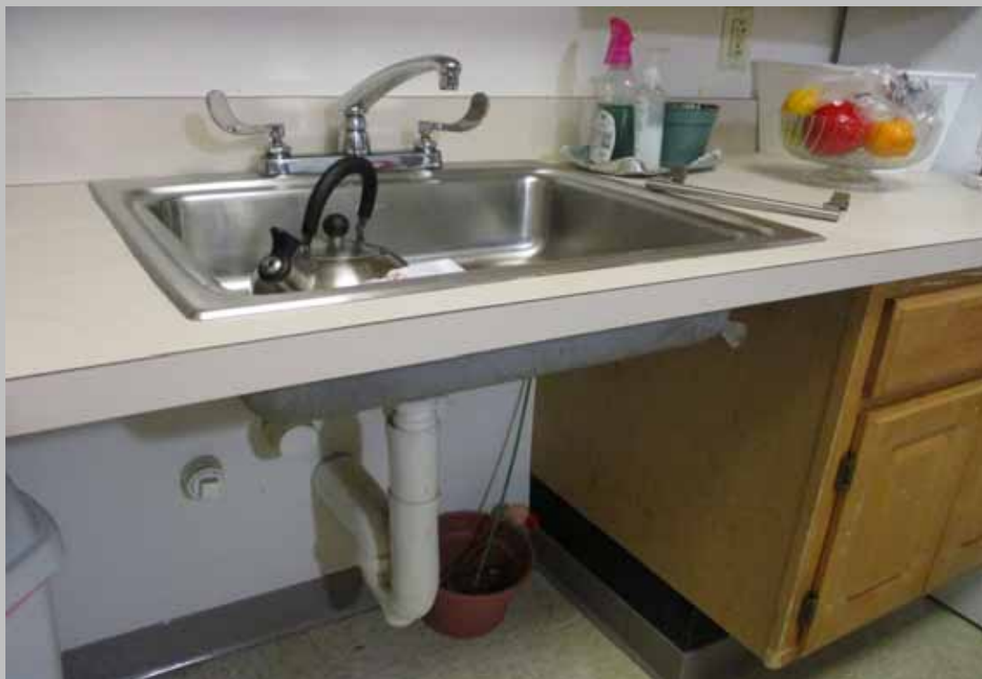
Correct scald proof piping in Unit 227.
