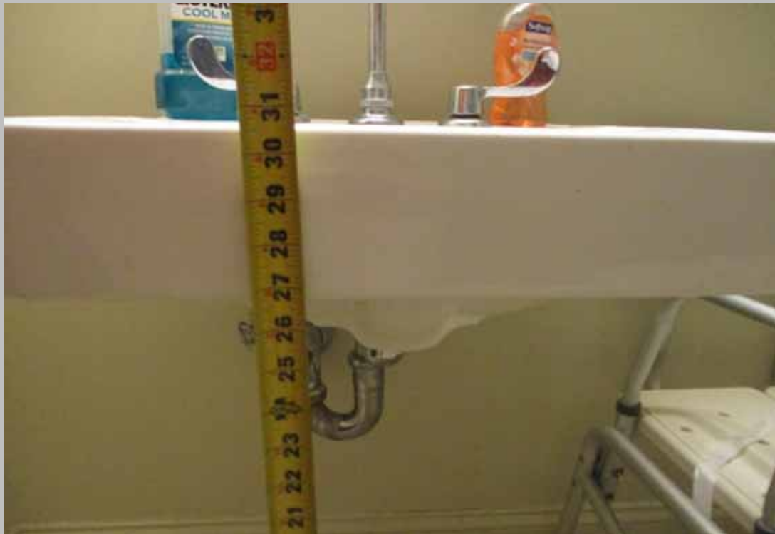
Bathroom sink height, levered hardware, missing scald proof piping Unit 221.
