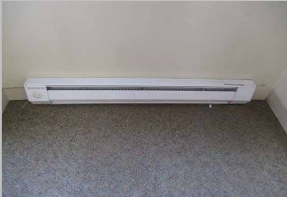
Typical floor-mounted electric space heater in stairwells.
