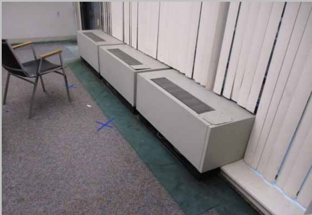
Fan coil units in common areas.
