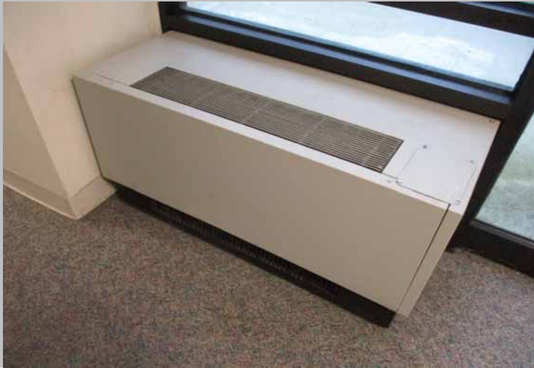
A fan coil unit in hallway.
