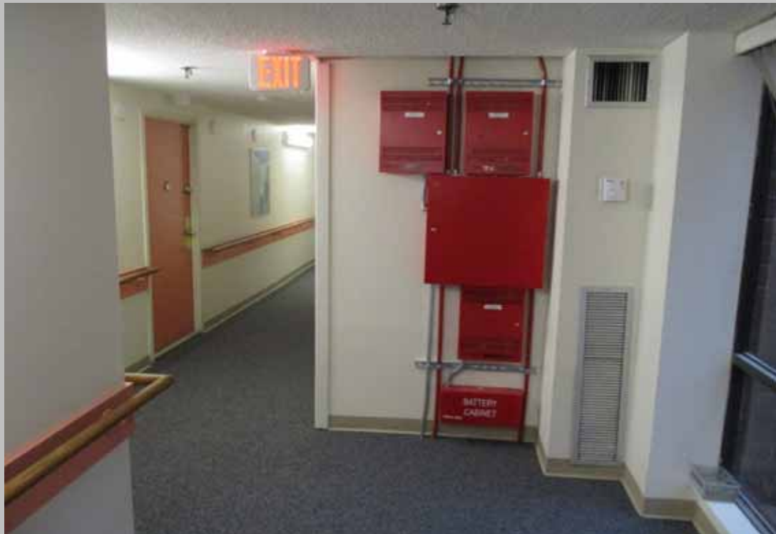
Booster fire panels in hallway.
