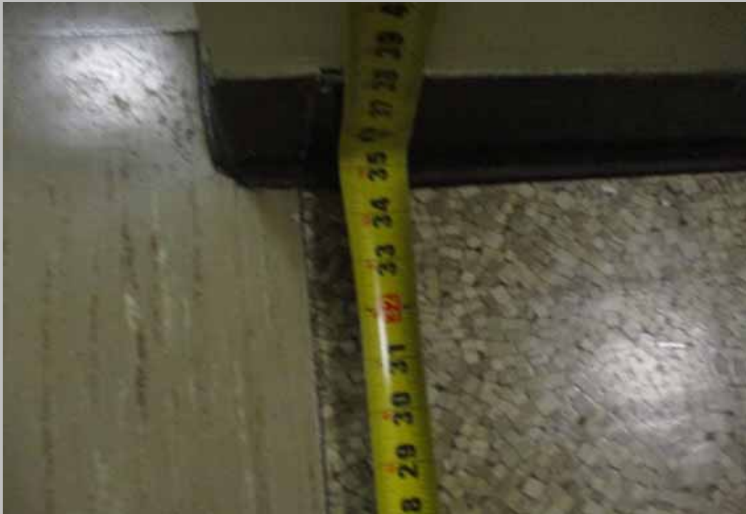
Correct kitchen entry width.
