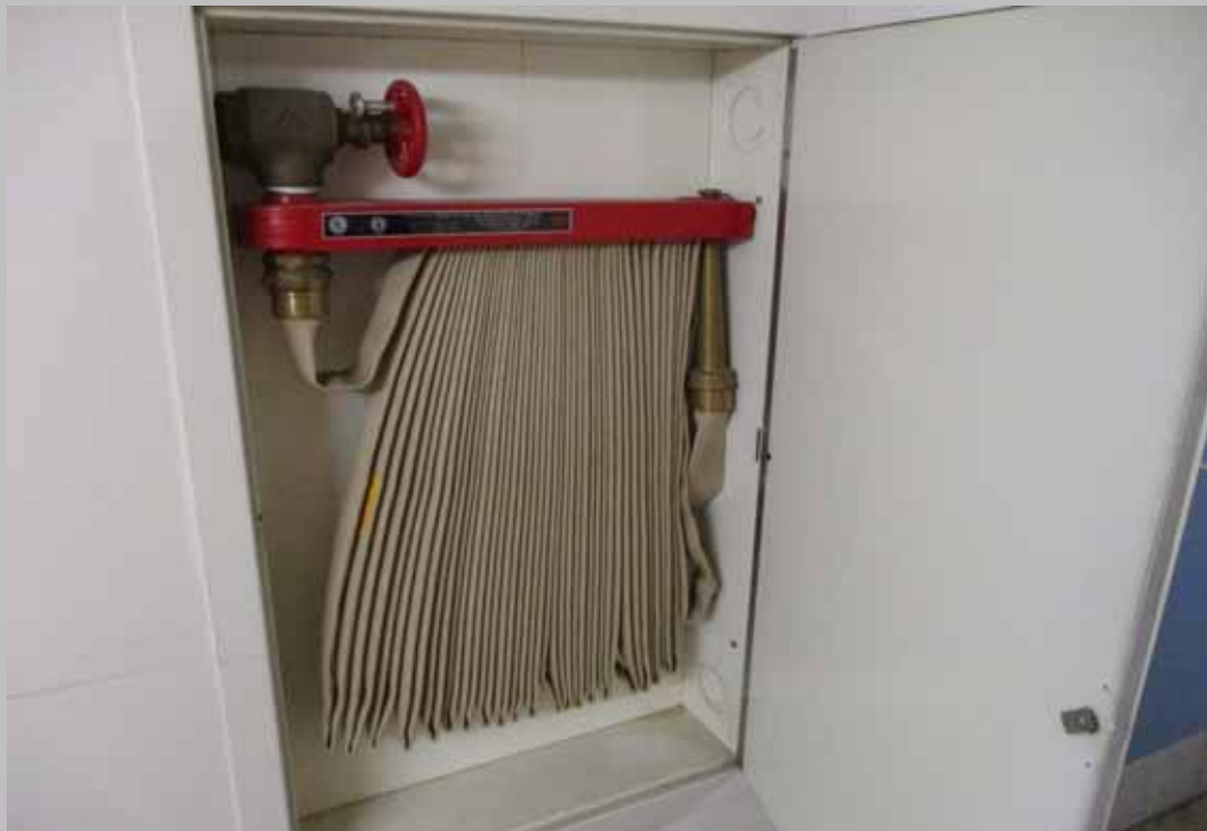
Fire hoses in hallways.
