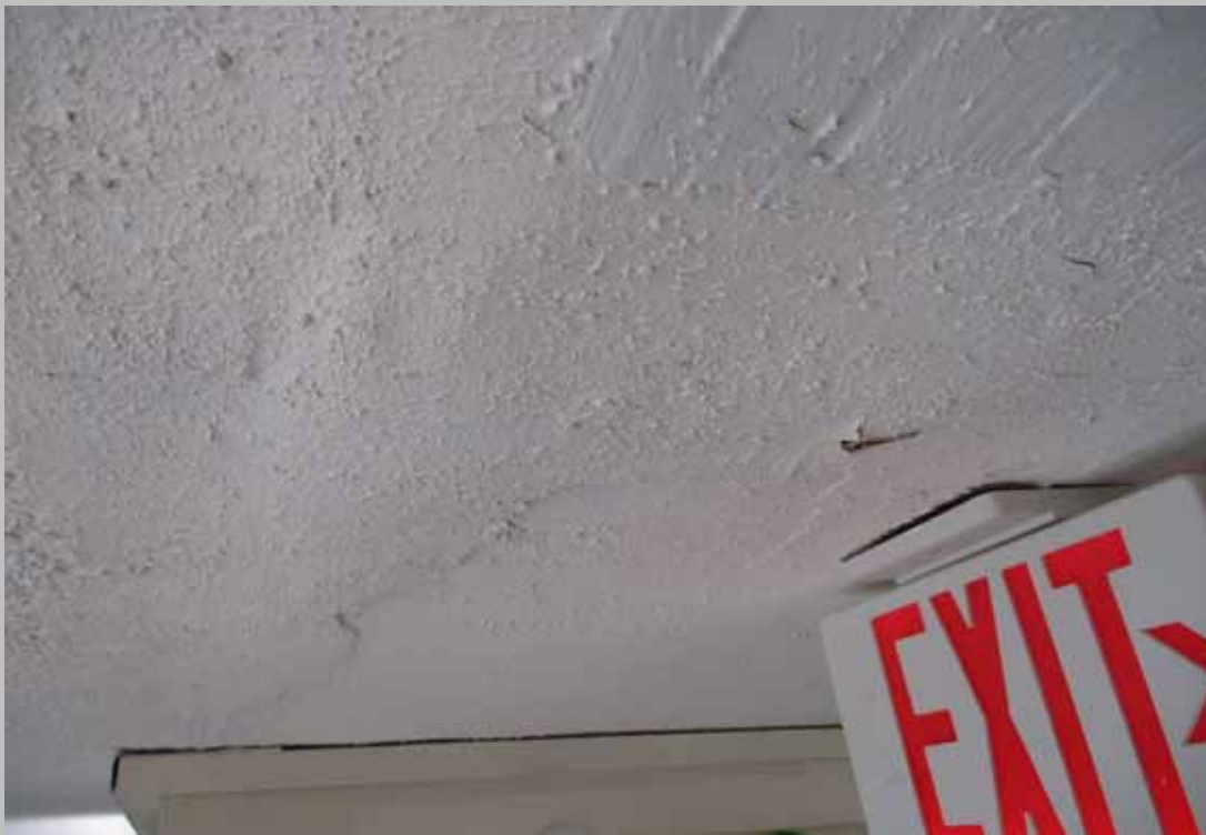
Evidence of recent roof leak and multiple repairs 5 th floor corridor.
