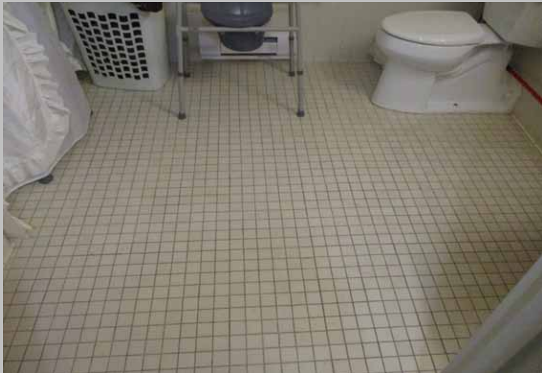
Proper clear floor space in bathroom of Unit 227.
