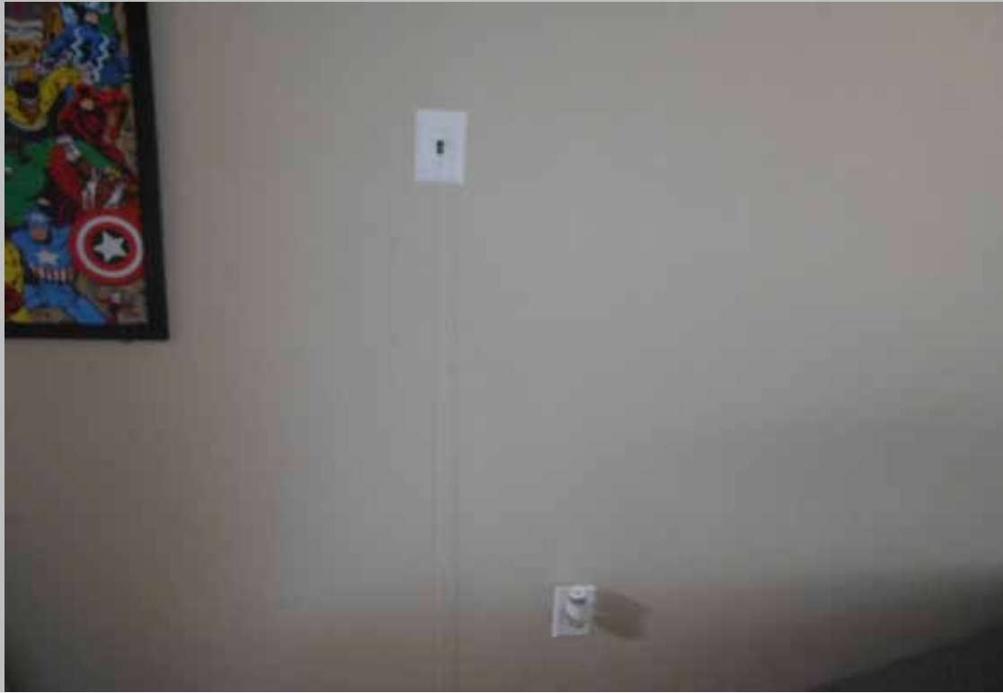
Typical emergency call pull cord (dwelling unit bedrooms and bathrooms)
