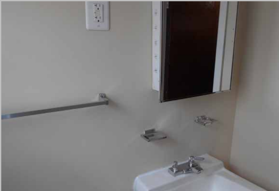
Typical GFCI outlet (dwelling unit kitchens and bathrooms)
