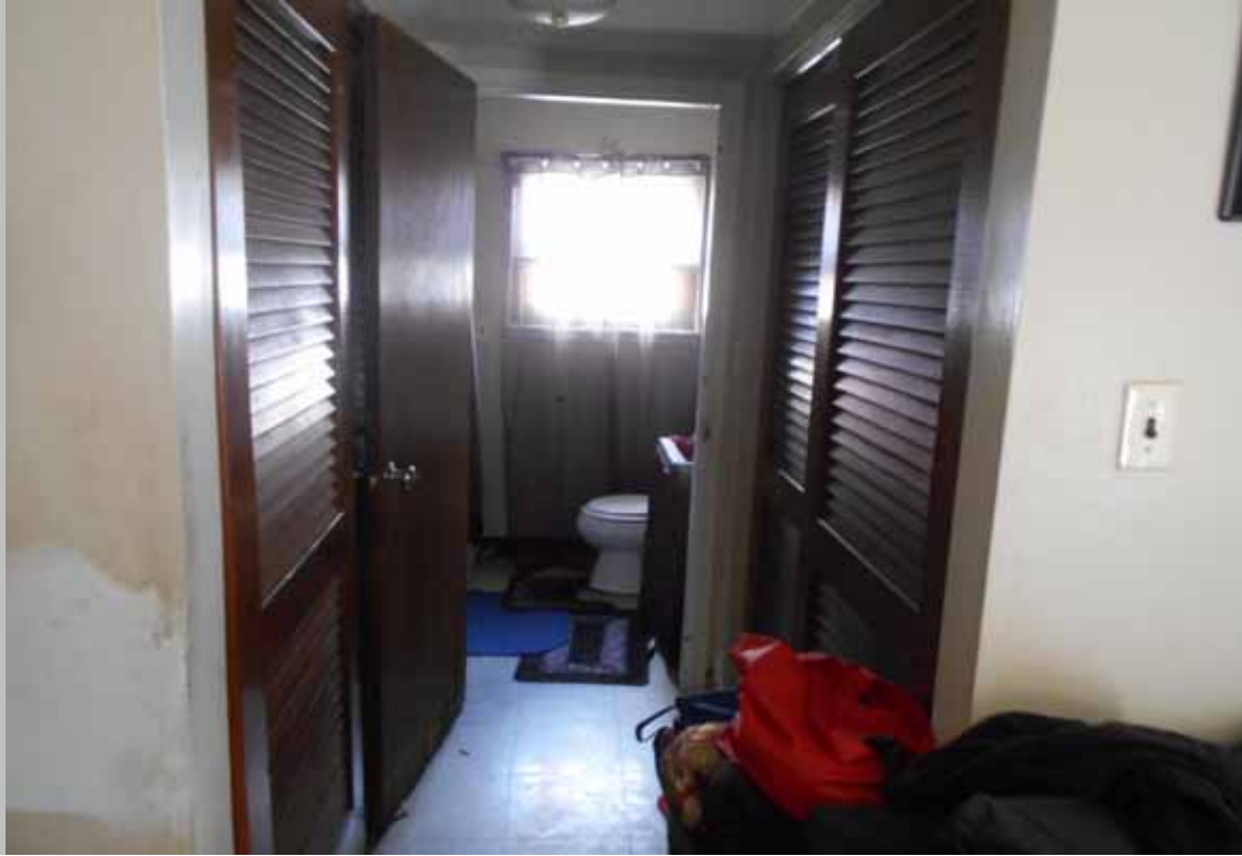
Missing paint along drywall - dwelling unit 25/47 Washington Street (Non-Critical Repair)
