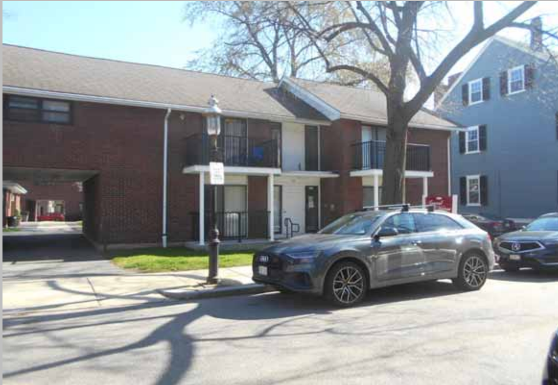
Primary entrance to leasing/management office - not connected to the accessible route (the rear entrance to the building is connected to the accessible route)
