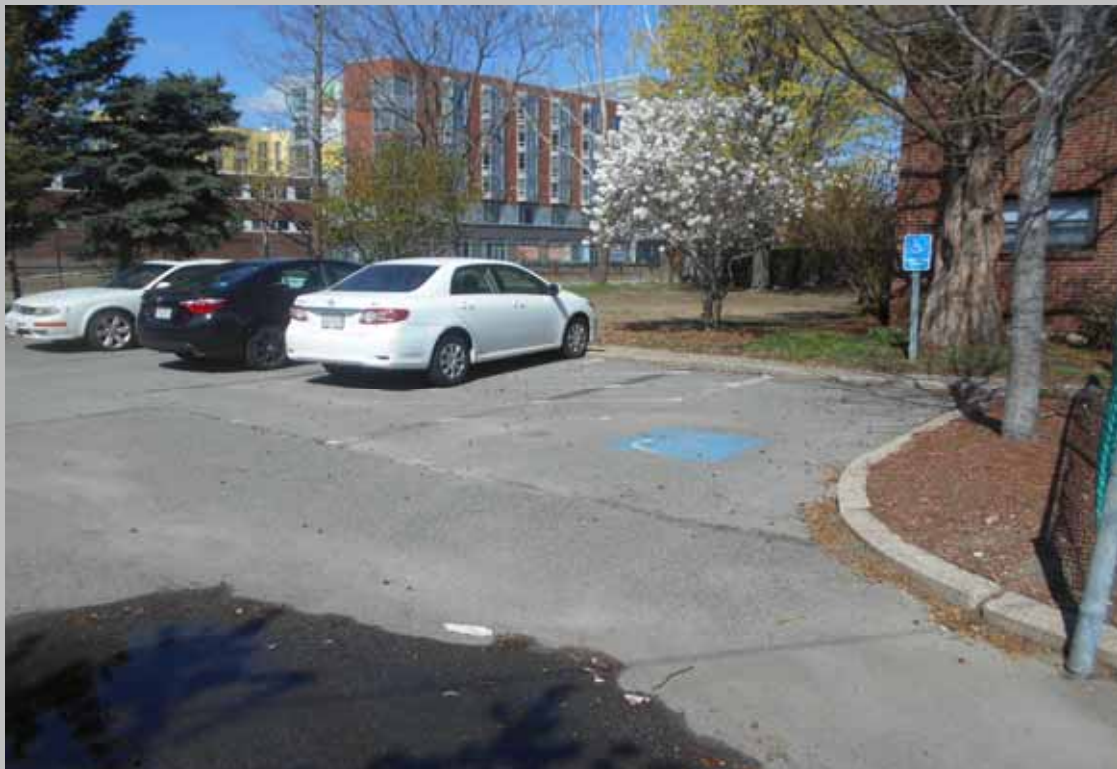
Parking lot missing a van-accessible handicapped parking space (Non-Compliant, ADA) – Critical Repair
