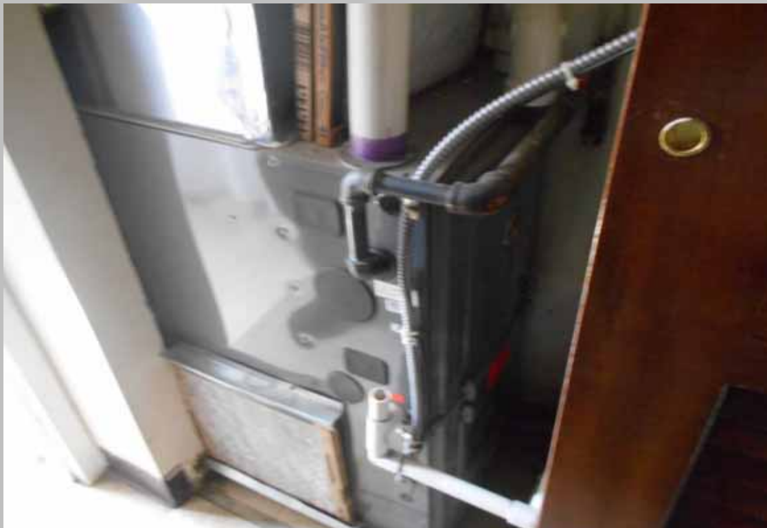
Typical gas furnace (dwelling units)
