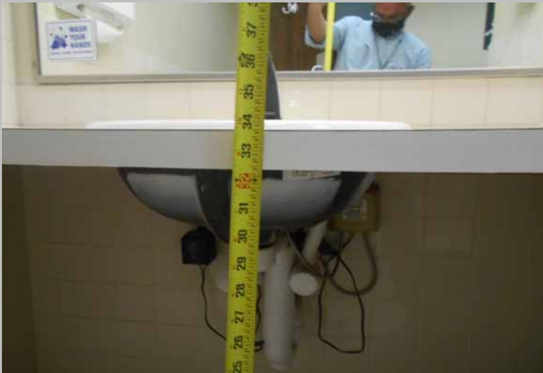
Restroom sink mounted at required 34-inches from floor – common area public unisex restroom (Compliant, UFAS)
