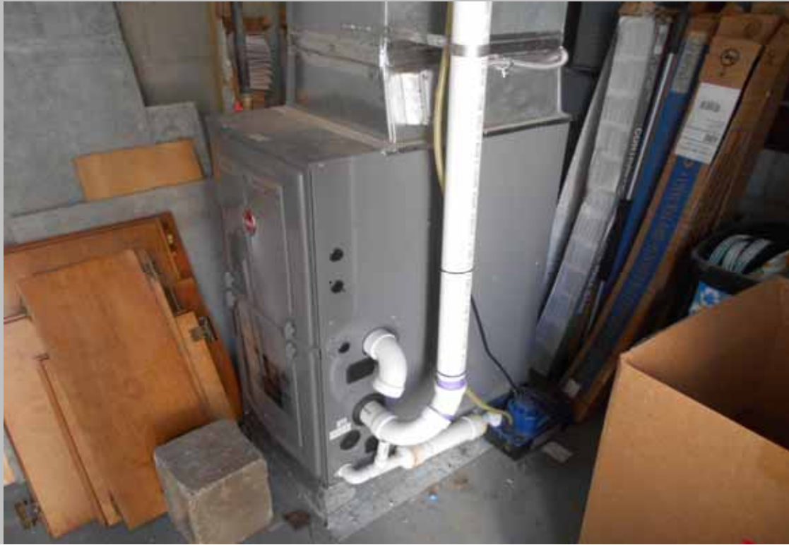
Typical gas furnace (Community Centers)
