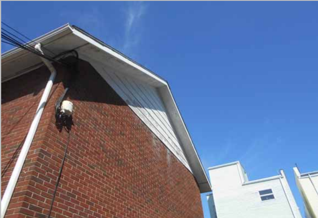
Example of siding in need of re-painting – 26 Union Street (Non-Critical Repair)
