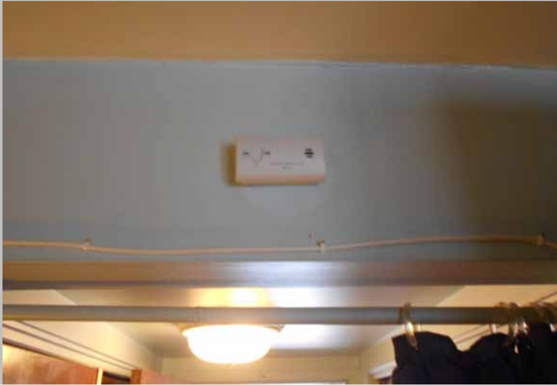
carbon monoxide detector (dwelling units)
