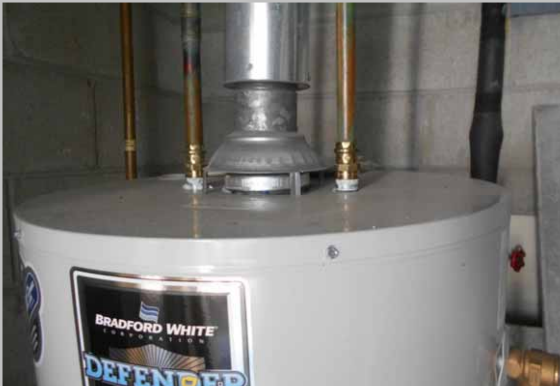
Typical gas-fired water heater (Community Centers)
