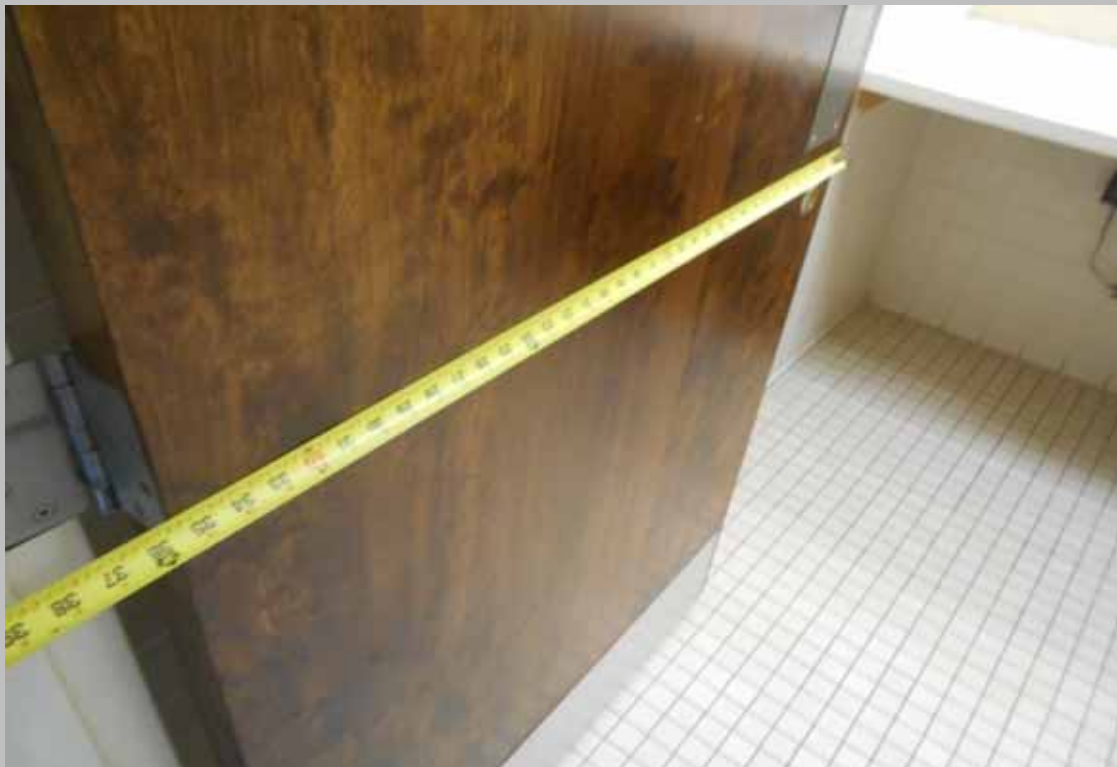
Sufficient clear door opening of at least 32-inches – common area public unisex restroom (Compliant, UFAS)
