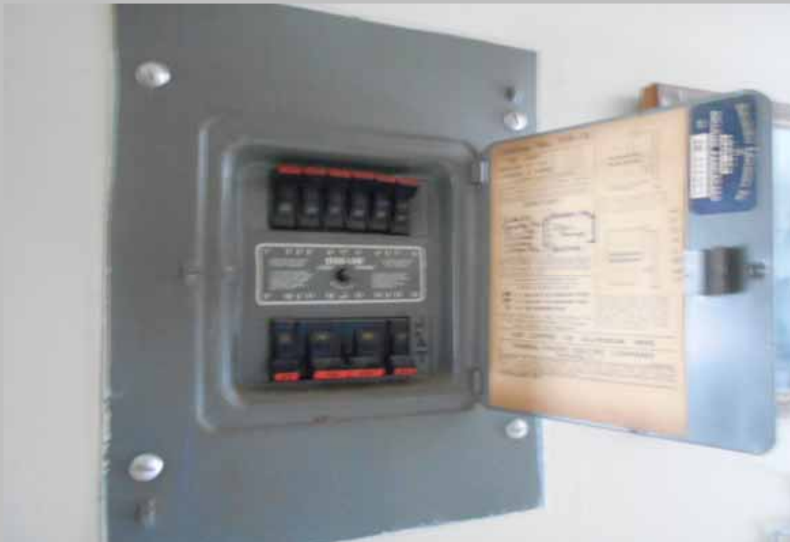
Federal Pacific Stab-Lok electric breaker panel - install new brand upon replacement (dwelling units)
