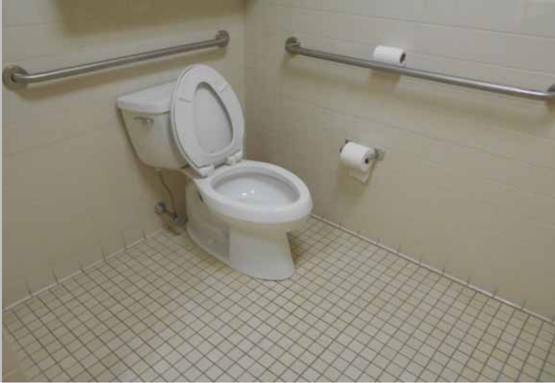
Side and rear grab bars at toilet – common area public unisex restroom (Compliant, UFAS)
