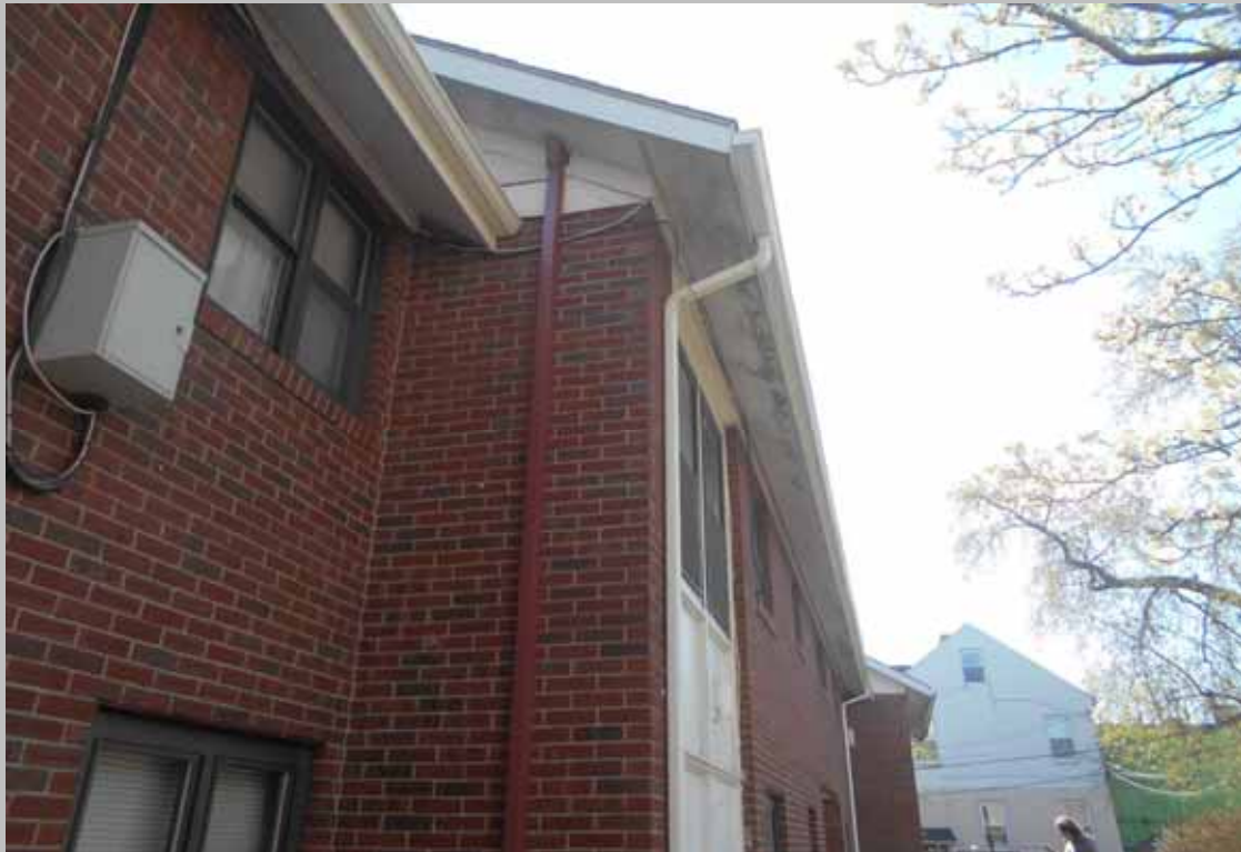
Example of a building exterior with mildew growth in need of pressure washing (Non-Critical Repair)
