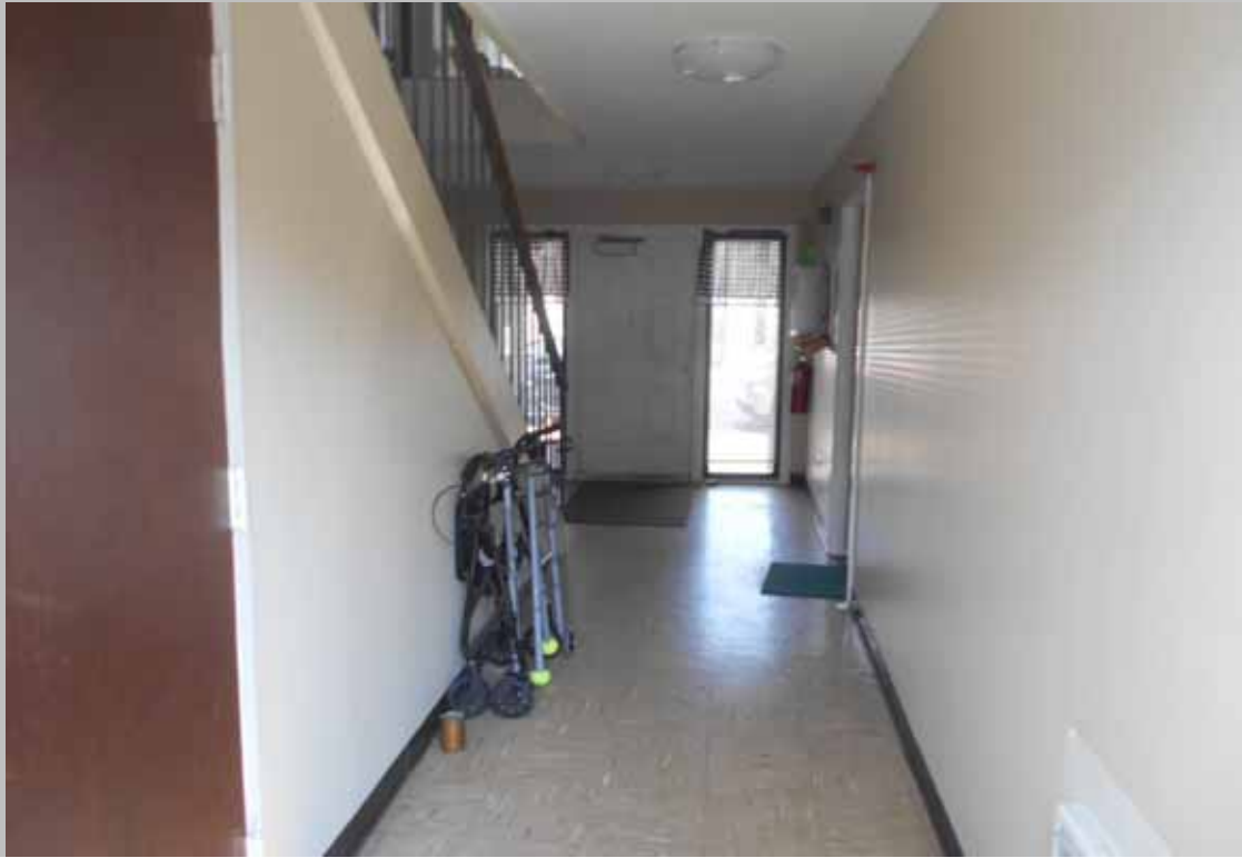
Typical fire extinguisher (common hallways)
