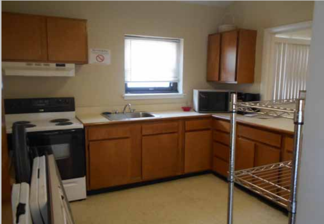
Community kitchen (Community Center 1) - lacking a front controlled range/oven unit, roll-under access at the sink, and lowered upper cabinetry
