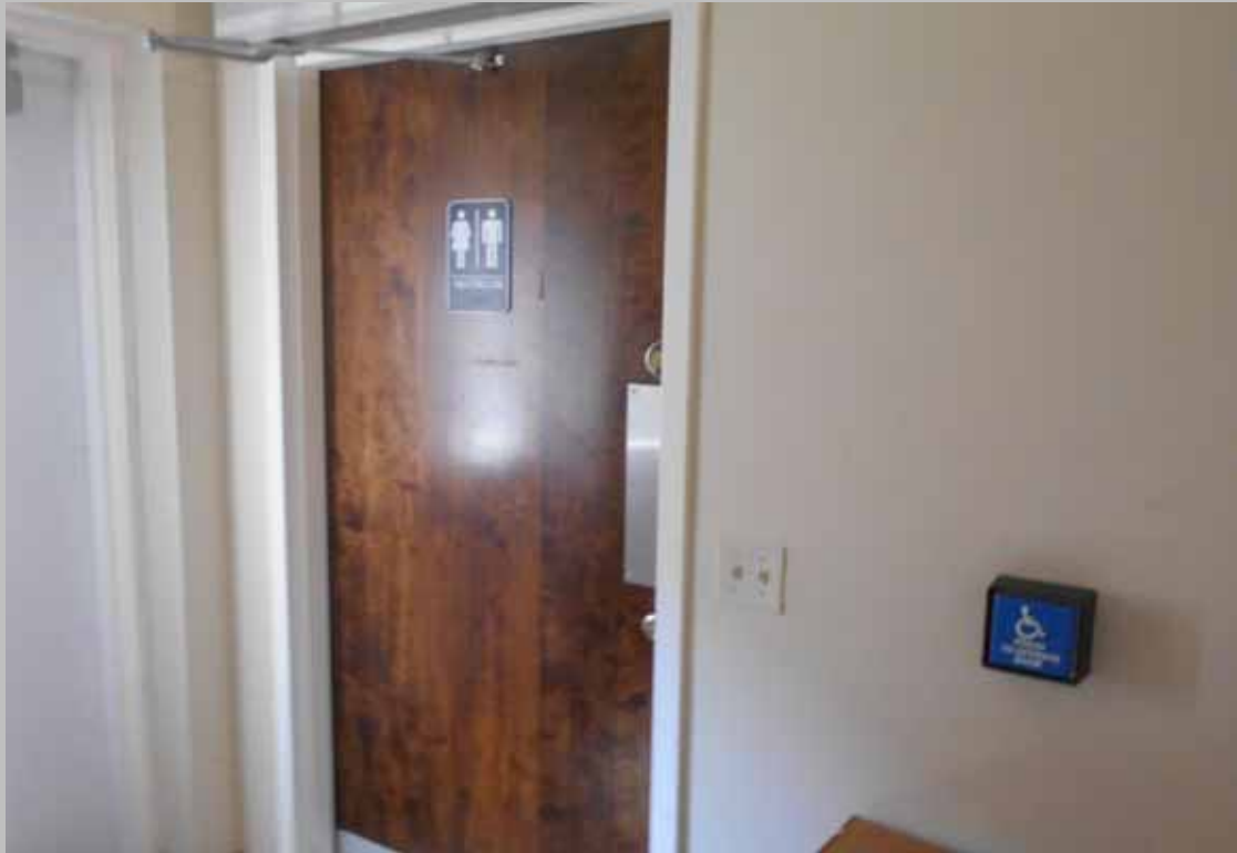
Accessible automatic door – common area public unisex restroom (Compliant, UFAS)
