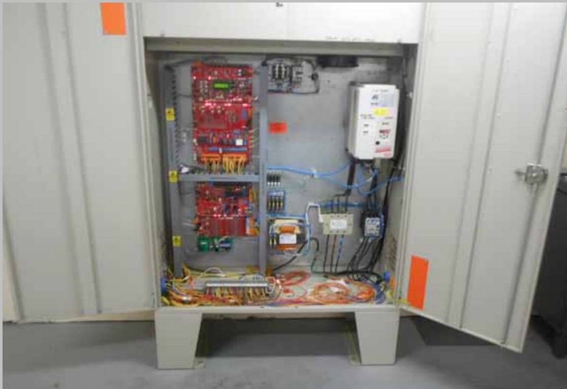
View of elevator equipment
