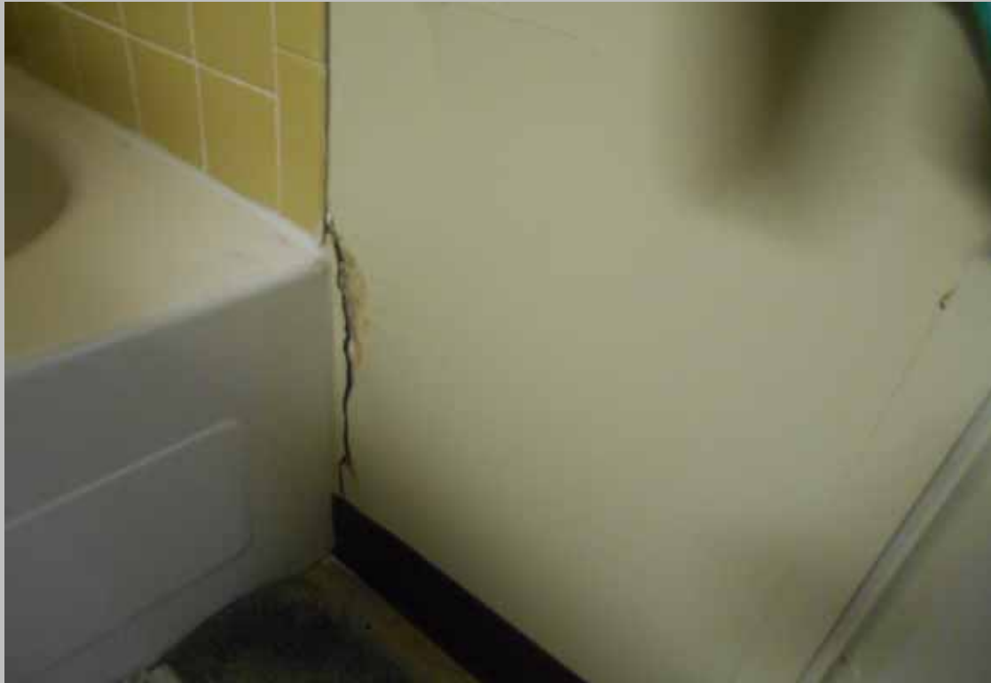
View of the damaged bathroom wall within dwelling unit 511 (Non-Critical Repair)
