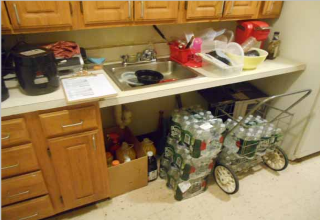
View of the roll-under kitchen sink within designated handicapped Unit 807 featuring non-compliant hardware and partial scald and abrasion protection
