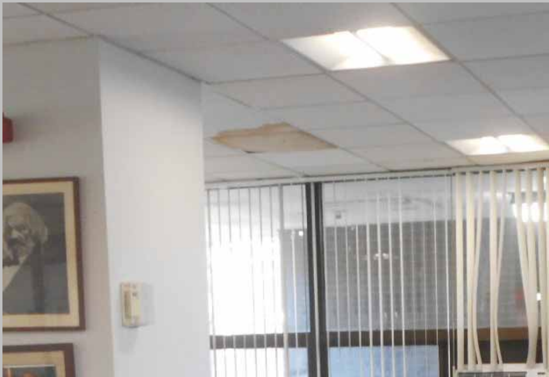
View of the water stained ACT in the common area sitting area (Non-Critical Repair)
