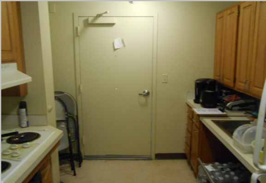
View of the entry door area within designated handicapped Unit 807 featuring levered handle door hardware
