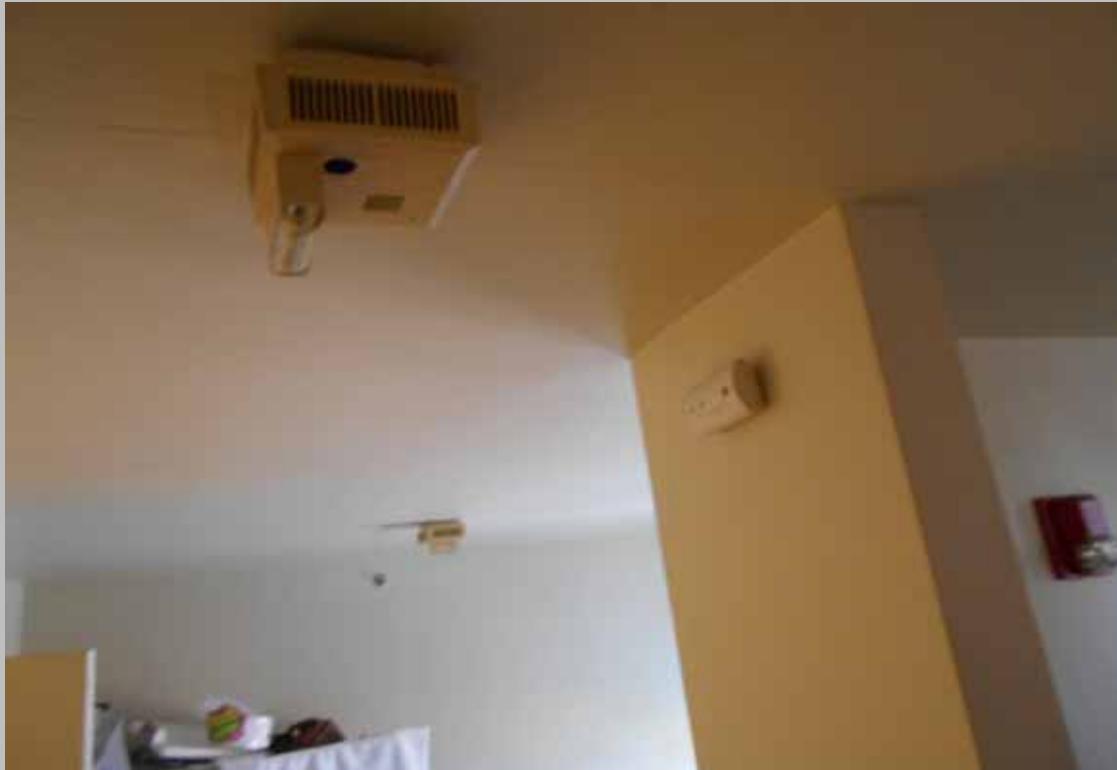
View of an A/V alarm and a carbon monoxide detector – dwelling unit
