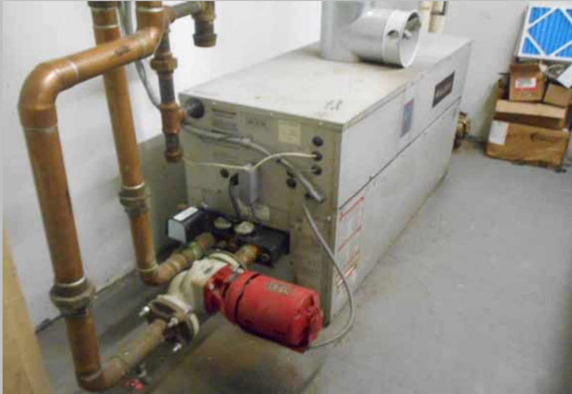
View of the DHW boiler
