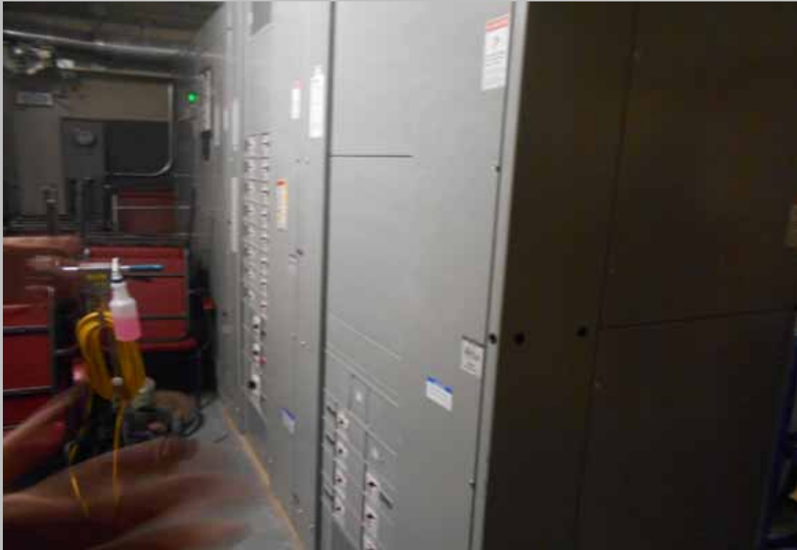
View of the switchboard
