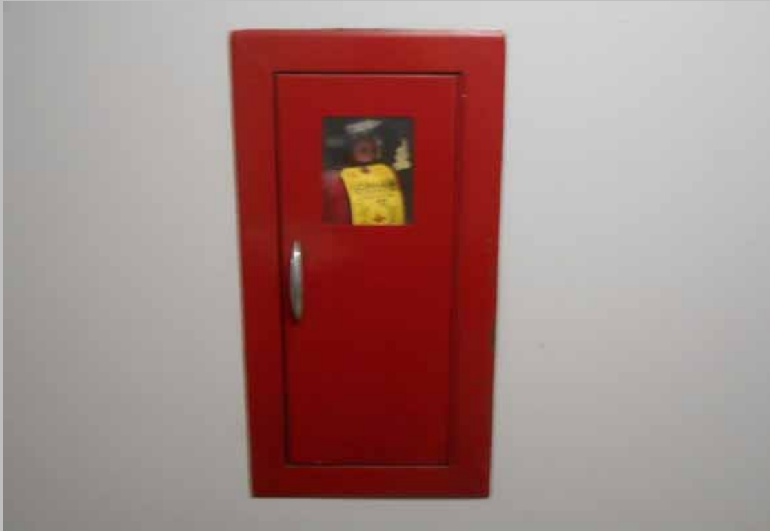
View of a fire extinguisher
