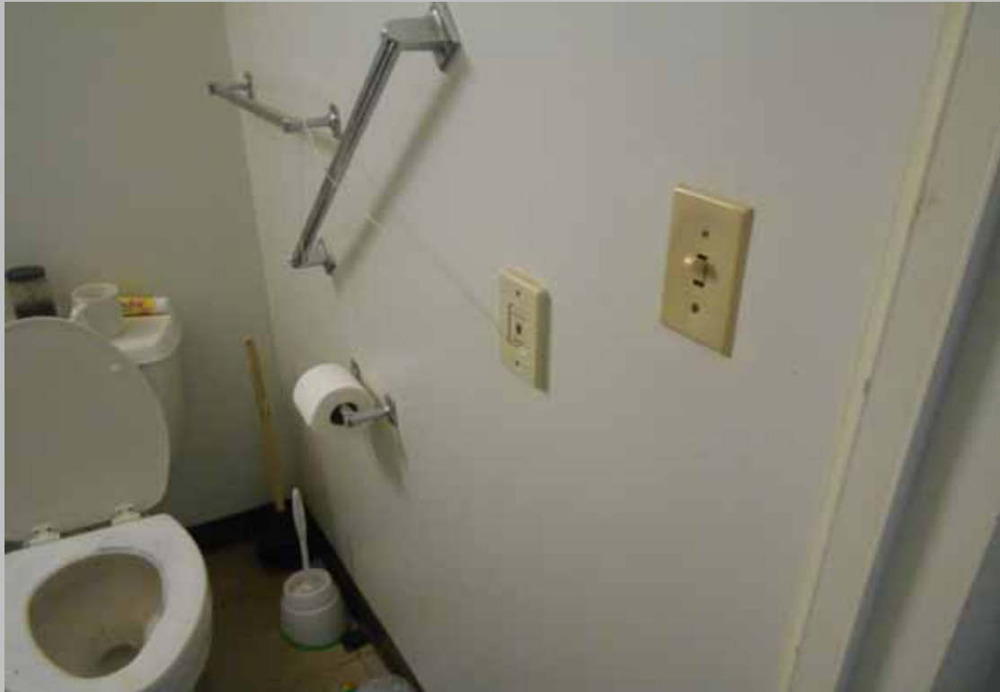
View of emergency pull cord – dwelling unit
