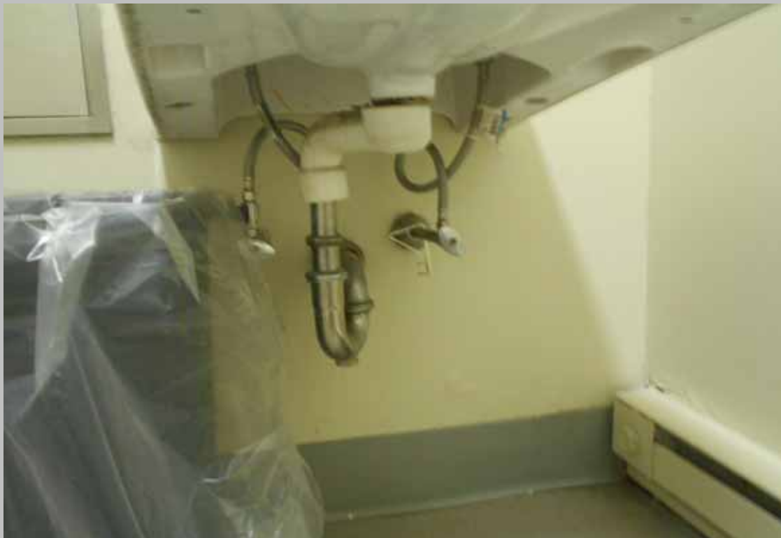
The common area Men's restroom sink is missing scald and abrasion protection at the under-sink plumbing (Critical Repair)
