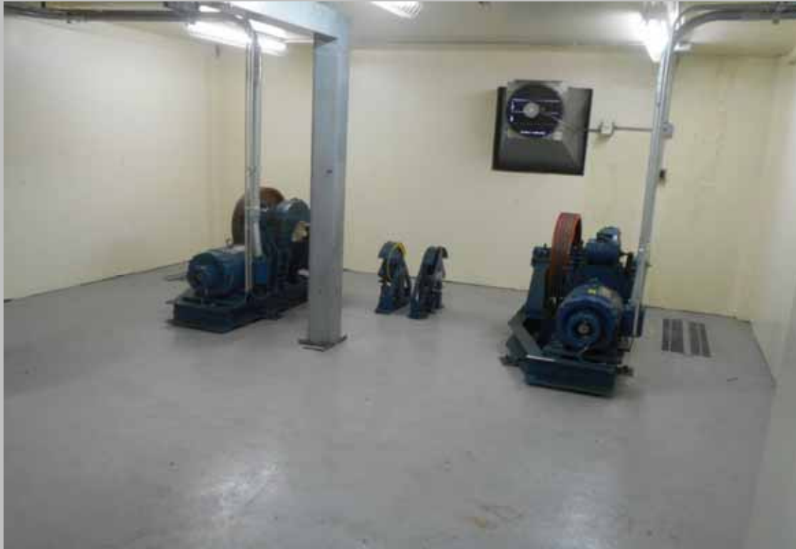
View of elevator equipment
