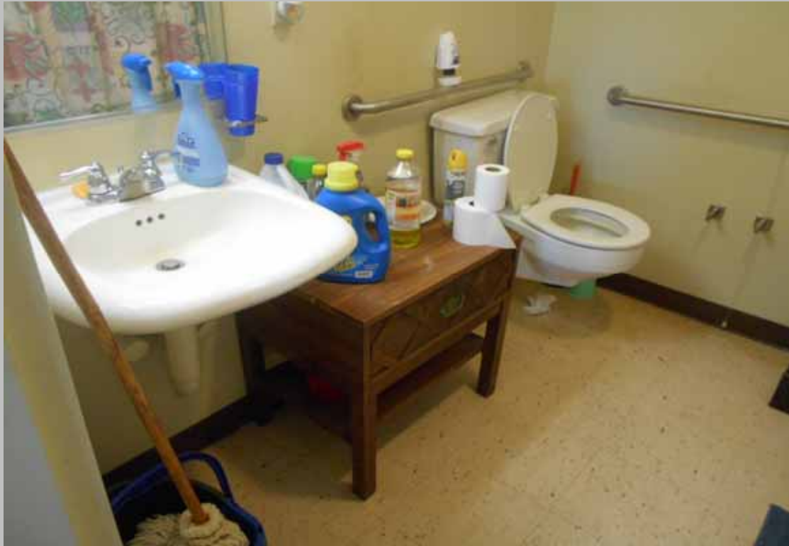
View of the bathroom within designated handicapped Unit 807 featuring compliant levered hardware, scald and abrasion protection, clear floor space, and toilet grab bars
