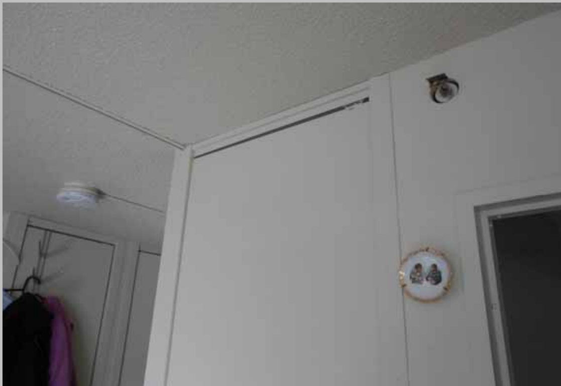
View of fire sprinkler head – dwelling unit
