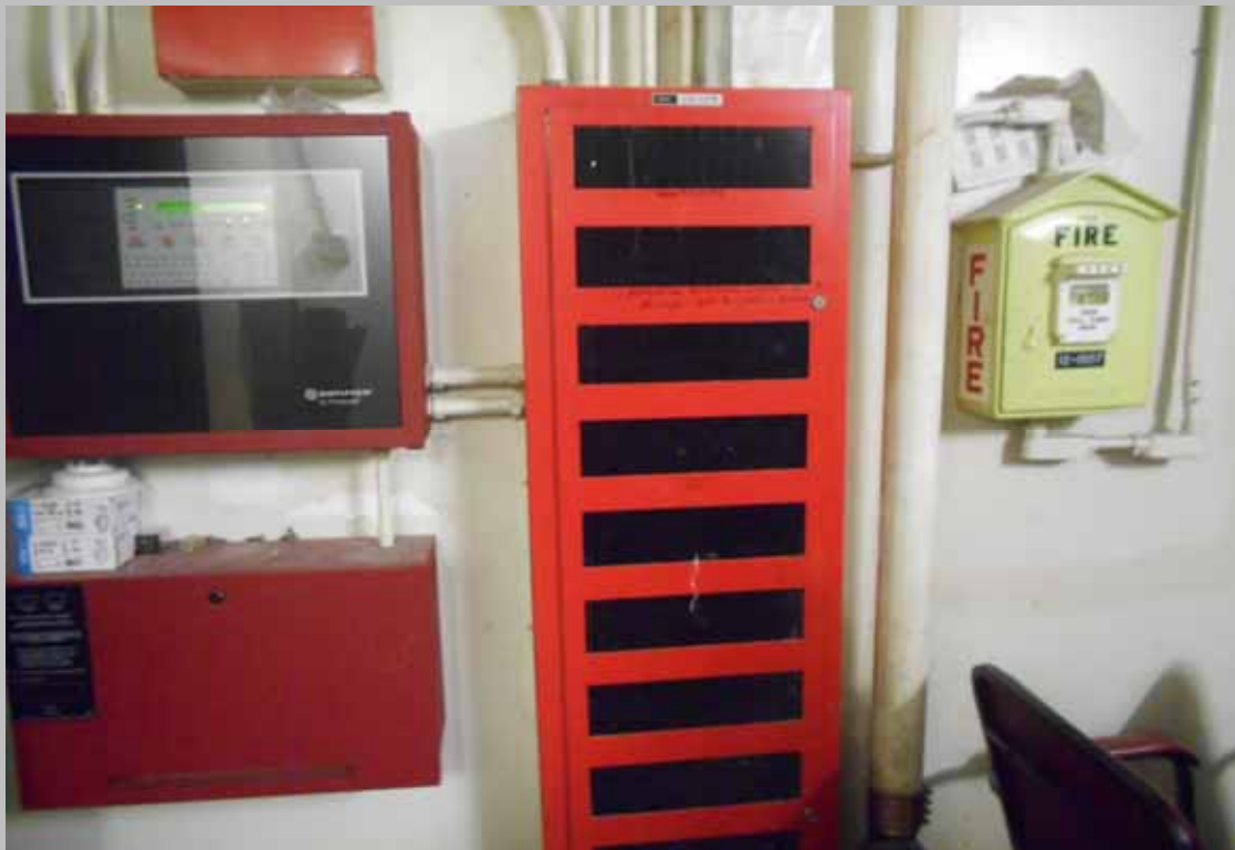
View of fire alarm control panel
