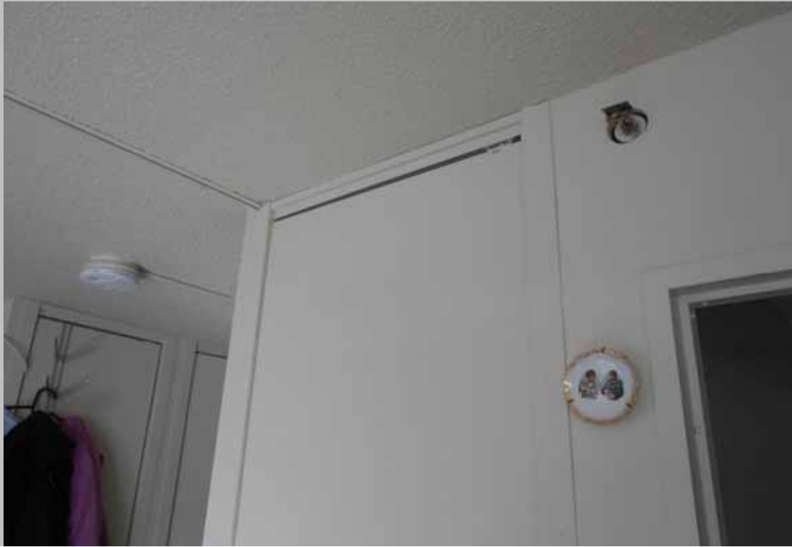
Dwelling unit 711 is missing an escutcheon plate at the sprinkler head above the bathroom door (Critical Repair)
