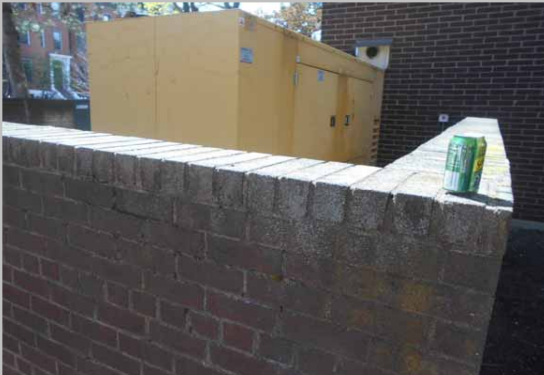
View of the generator
