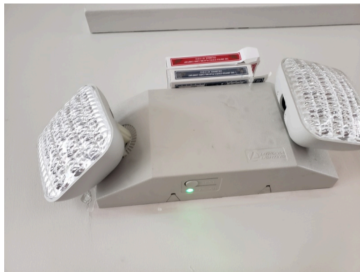
Life & Fire Safety: Typical emergency lighting found throughout the site.
