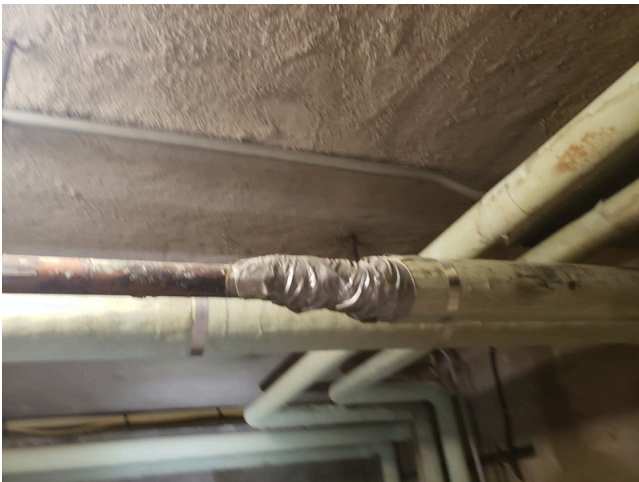
31. Plumbing: Typical corroded pipes found throughout the property. (Non-Critical Repair)
