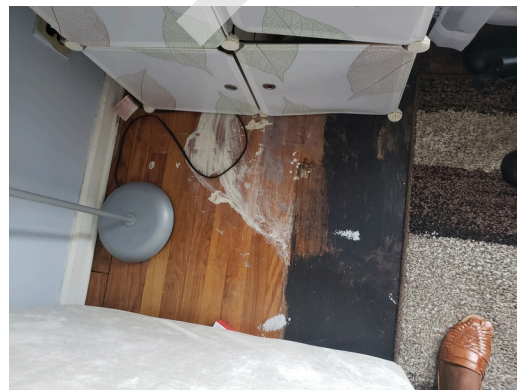
Dwelling Unit Interior Elements: Damaged finishes observed in unit 4. (Non-Critical Repair)
