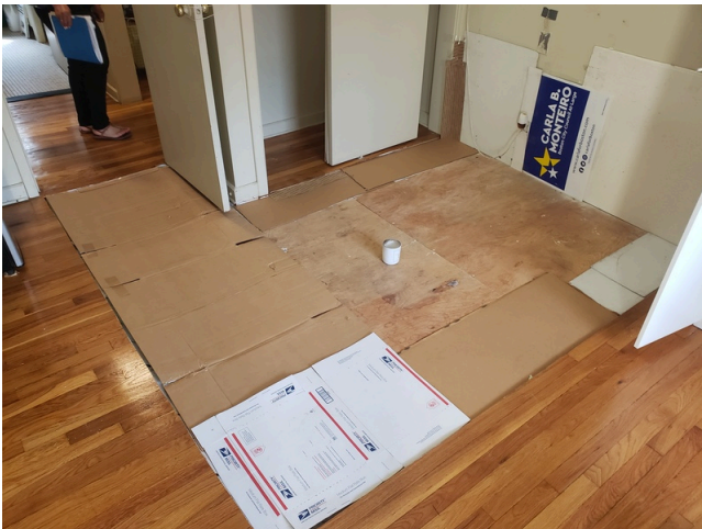
19. Building 2; Unit: 35; Floor: 2; Style: 1 Bed / 1 Bath: Living room with missing finishes. (Critical Repair)
