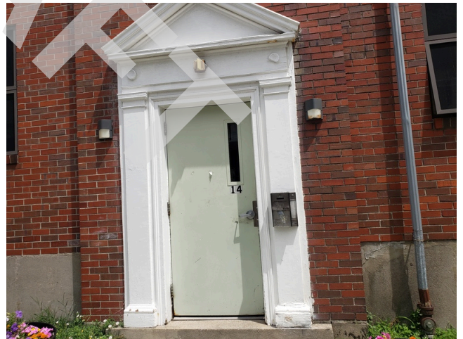
40. Exterior Doors & Entry Systems: Typical building access door found throughout the site.
