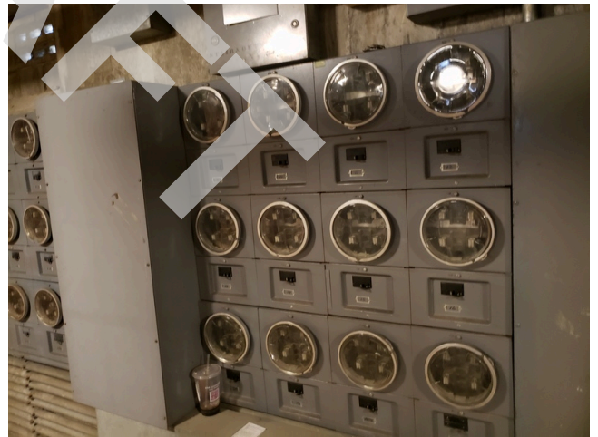
88. Electrical System: Typical electric meter bank found throughout the site.
