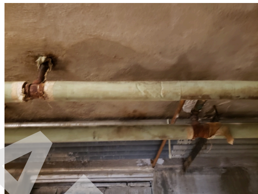
Plumbing: Typical corroded pipes found throughout the property. (Non-Critical Repair)
