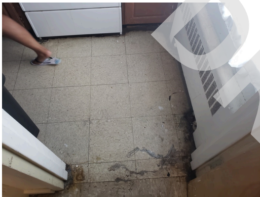
Dwelling Unit Interior Elements: Damaged finishes observed in unit 4. (Non-Critical Repair)
