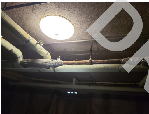
Plumbing: Typical corroded pipes found throughout the property. (Non-Critical Repair)
