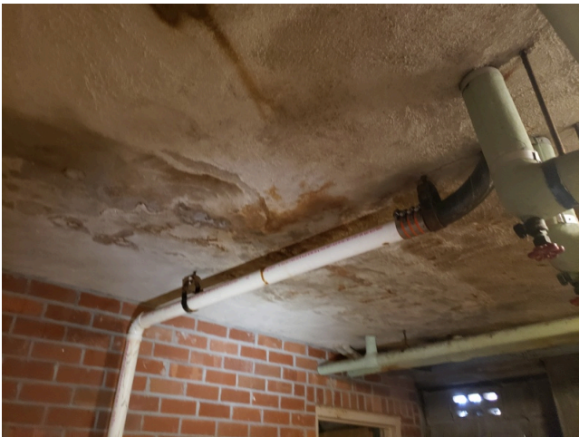
75. Plumbing: Typical cast iron and PVC waste pipes found throughout the property.
