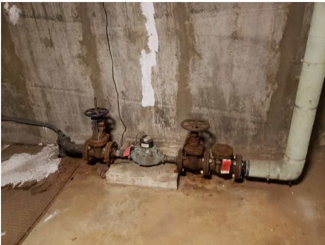
27. Site Utilities: Central water meter found at the site.
