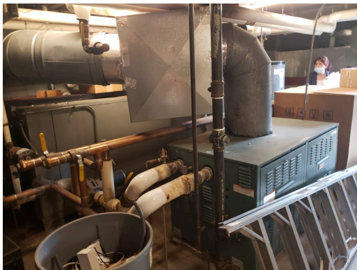
Central gas boilers found on the property.
