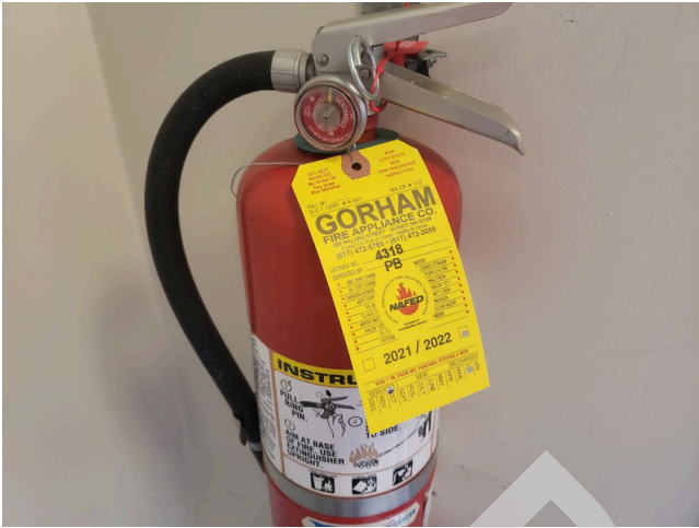
97. Life & Fire Safety: Typical fire extinguisher found throughout the site.
