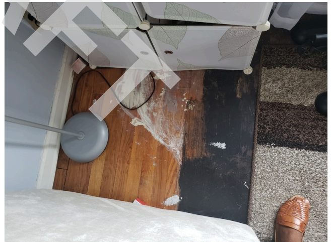
112. Dwelling Unit Interior Elements: Damaged finishes observed in unit 4. (Non-Critical Repair)
