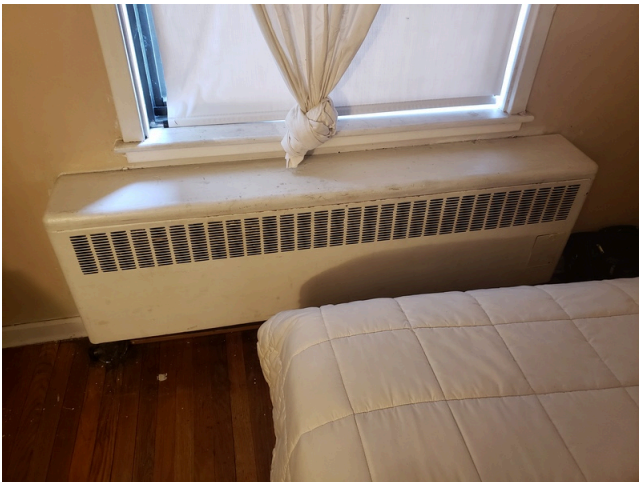
7. Building 1; Unit: 4; Floor: 2; Style: 2 Bed / 1 Bath: Heater.
