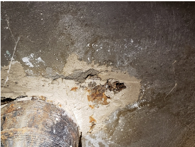
35. Foundation: Typical cracks on basement walls and ceilings found throughout the site. (Critical Repair)
