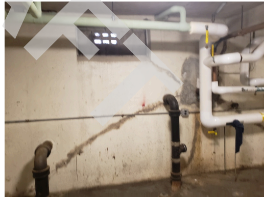
Foundation: Typical cracks on basement walls and ceilings found throughout the site. (Critical Repair)
