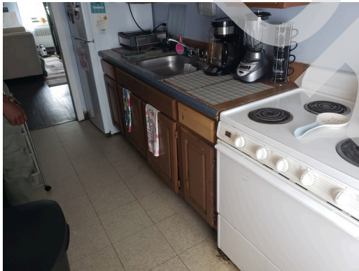
Cabinets & Fixtures: Typical dwelling unit kitchen sink, countertop, and wood cabinets found throughout the site.
