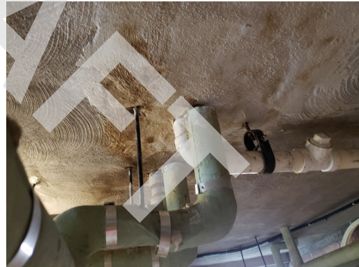
Plumbing: Typical cast iron and PVC waste pipes found throughout the property.
