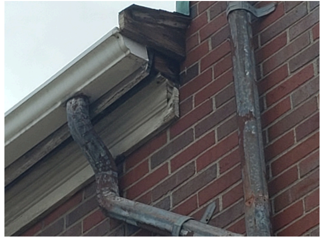
46. Sidewall System: Typical weathered and damaged wood trim found throughout the site. (Non-Critical Repair)
