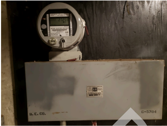
89. Electrical System: Central electric meter found at the site.
