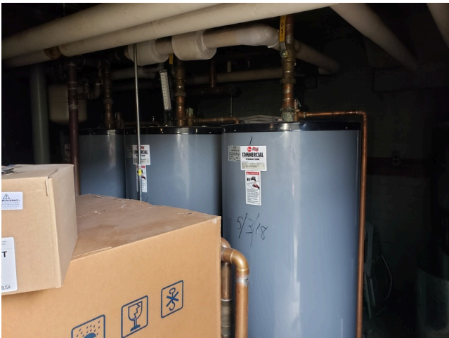
79. Plumbing: Storage tanks found on the property.
