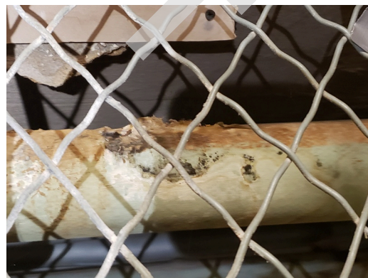
Moisture and Microbial Growth: Mold on water pipes observed throughout the site. (Critical Repair)
