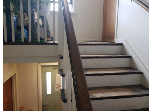
Common Area Interior Elements: Typical staircase with worn down finishes found throughout the site. (Non-Critical Repair)
