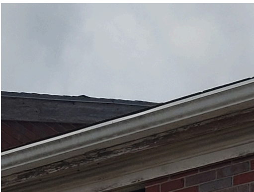
Sidewall System: Typical weathered and damaged wood trim found throughout the site. (Non-Critical Repair)
