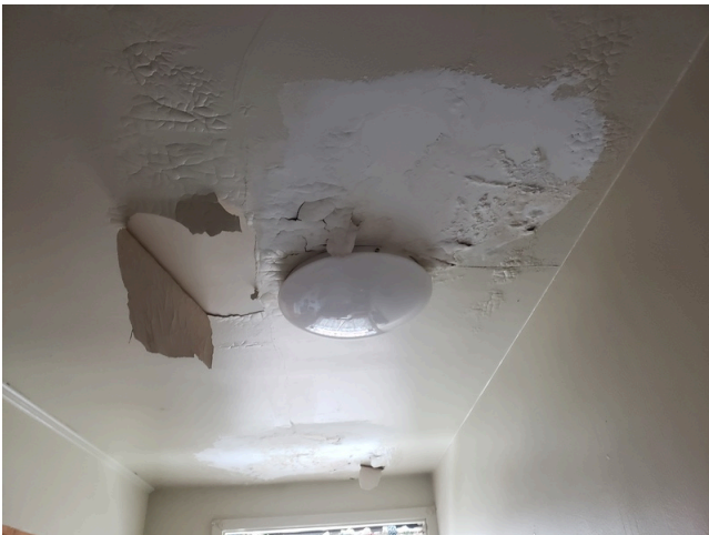
115. Dwelling Unit Interior Elements: Damaged finishes observed in unit 20. (Non-Critical Repair)
