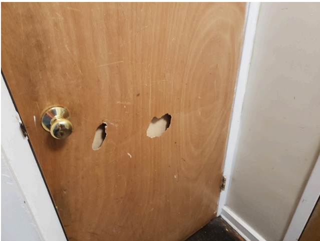
111. Dwelling Unit Interior Elements: Damaged finishes observed in unit 4. (Non-Critical Repair)
