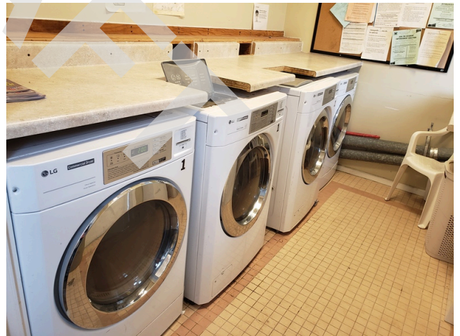
100. Common Area Interior Elements: Common laundry room.
