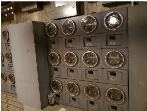
Electrical System: Typical electric meter bank found throughout the site.
