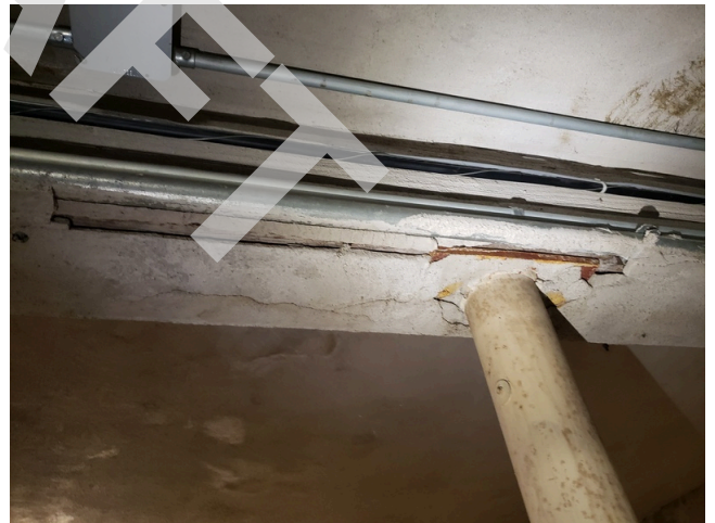
36. Foundation: Typical cracks on basement walls and ceilings found throughout the site. (Critical Repair)
