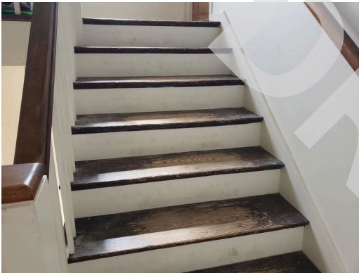
Common Area Interior Elements: Typical staircase with worn down finishes found throughout the site. (Non-Critical Repair)
