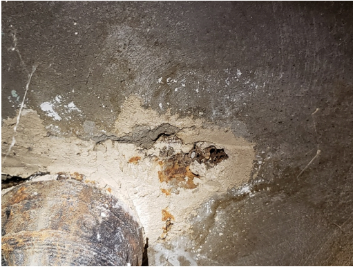
Foundation: Typical cracks on basement walls and ceilings found throughout the site. (Critical Repair)
