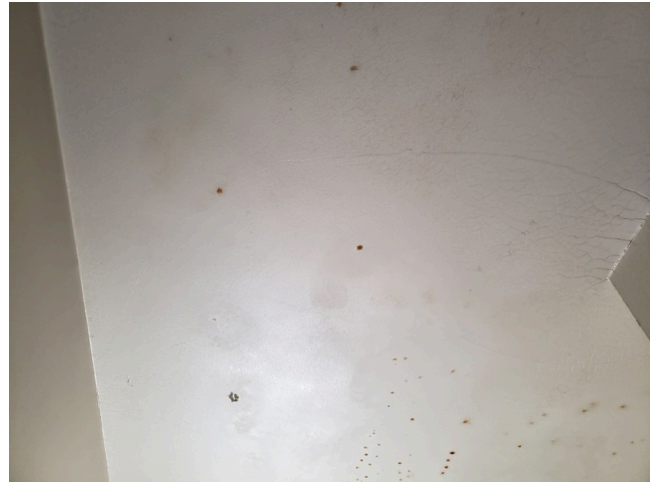
118. Dwelling Unit Interior Elements: Damaged finishes observed in unit 20. (Non-Critical Repair)
