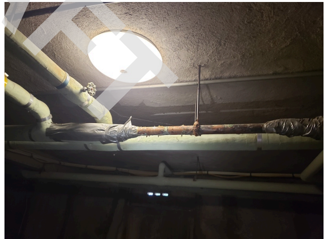
76. Plumbing: Typical corroded pipes found throughout the property. (Non-Critical Repair)
