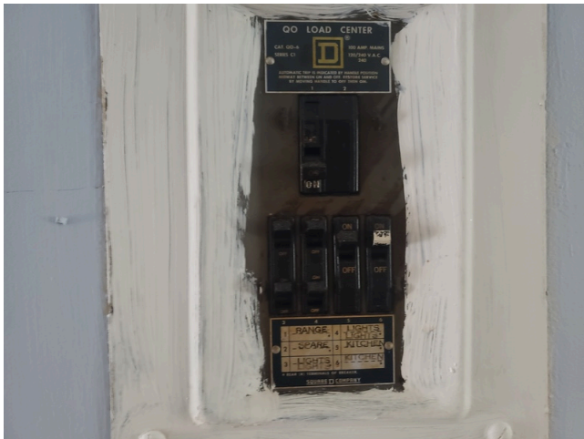
91. Electrical System: Typical dwelling unit electric panel found throughout the site.
