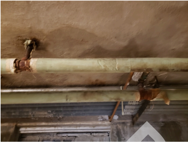
77. Plumbing: Typical corroded pipes found throughout the property. (Non-Critical Repair)
