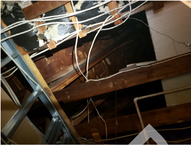
121. Dwelling Unit Interior Elements: Typical damaged sheetrock ceilings found throughout the site. (Non-Critical Repair)
