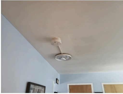
Life & Fire Safety: Typical non-compliant smoke detector found throughout the site. (Critical Repair)
