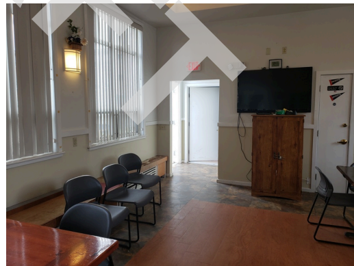
Life & Fire Safety: Typical illuminated exit sign found throughout the site.
