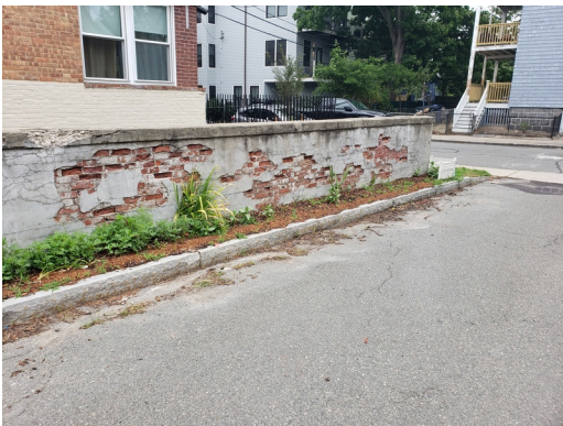
Landscaping & Appurtenances: Damaged CMU wall found on the north perimeter of the property. (Non-Critical Repair)
