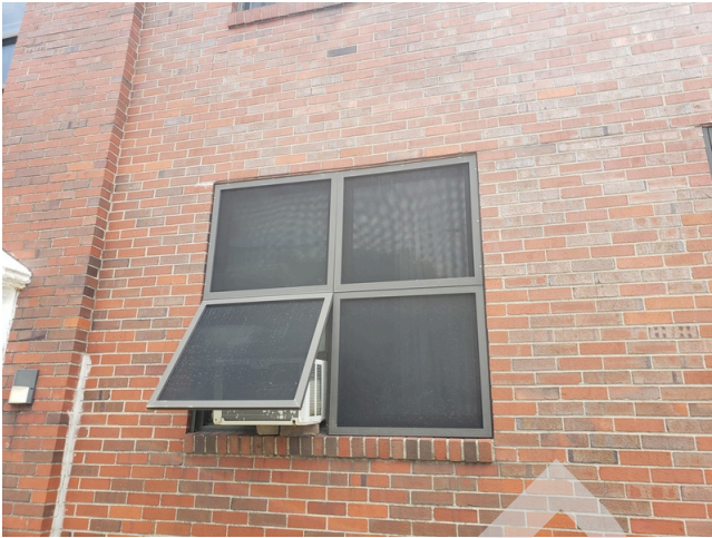
81. HVAC Systems: Typical tenant owned window unit AC system found throughout the site.
