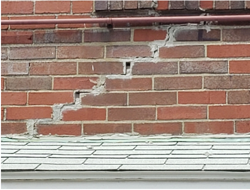
Sidewall System: Typical cracked unpainted brick found throughout the site. (Non-Critical Repair)
