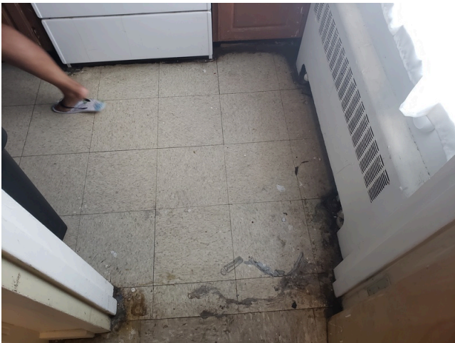
3. Building 1; Unit: 4; Floor: 2; Style: 2 Bed / 1 Bath: Damaged kitchen finishes. (Non-Critical Repair)
