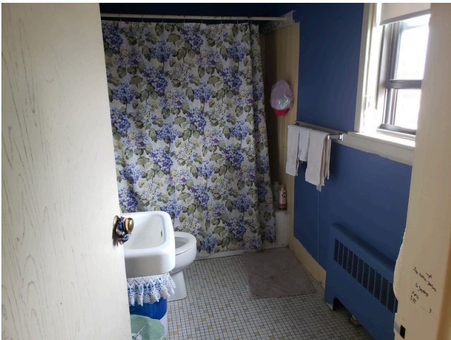
107. Dwelling Unit Interior Elements: Typical tile flooring and sheetrock finish found in dwelling units throughout the site.
