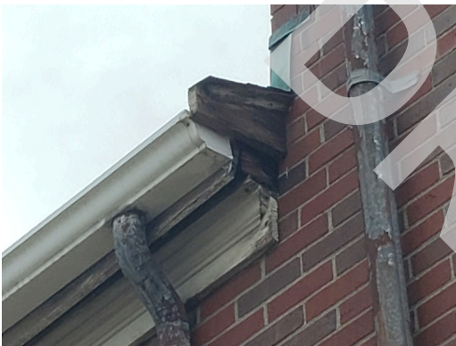
Sidewall System: Typical weathered and damaged wood trim found throughout the site. (Non-Critical Repair)
