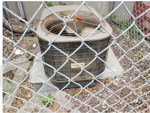
HVAC Systems: 3 ton AC system found at the community room.
