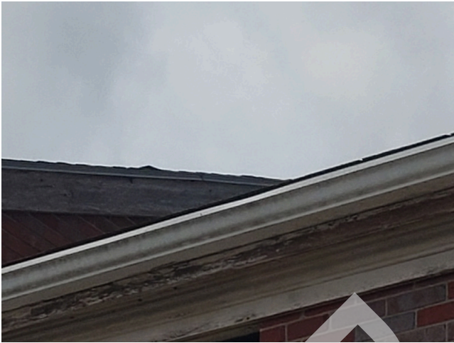
49. Sidewall System: Typical weathered and damaged wood trim found throughout the site. (Non-Critical Repair)
