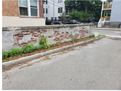
Landscaping & Appurtenances: Damaged CMU wall found on the north perimeter of the property. (Non-Critical Repair)
