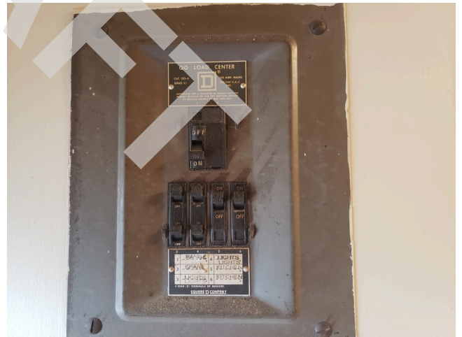
92. Electrical System: Typical dwelling unit electric panel found throughout the site.
