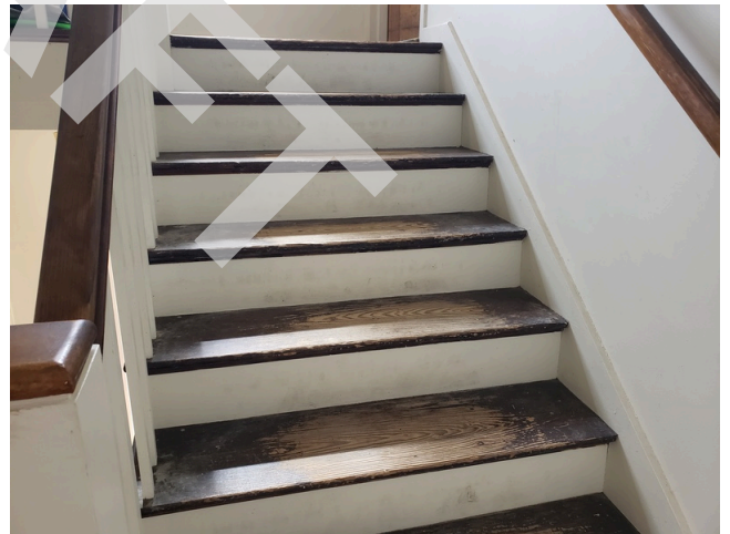
104. Common Area Interior Elements: Typical staircase with worn down finishes found throughout the site. (Non-Critical Repair)
