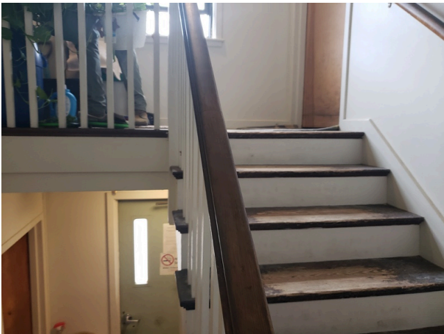
103. Common Area Interior Elements: Typical staircase with worn down finishes found throughout the site. (Non-Critical Repair)
