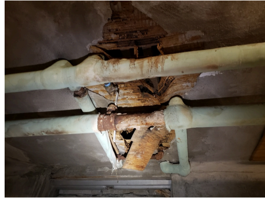
Foundation: Typical cracks on basement walls and ceilings found throughout the site. (Critical Repair)
