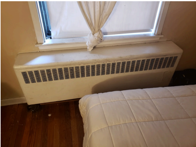
87. HVAC Systems: Typical hydronic radiant heater found in dwelling units throughout the property.
