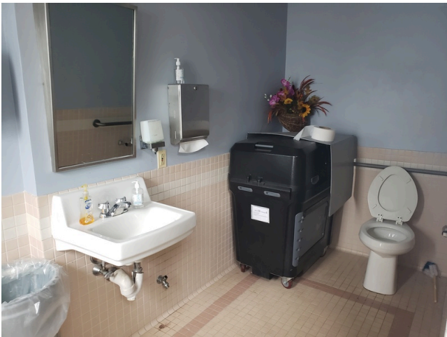
131. UFAS Concern: Common accessible restroom without levered sink hardware. (Critical Repair)
