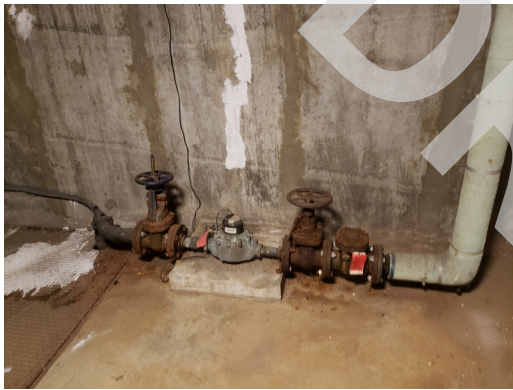
Site Utilities: Central water meter found at the site.
