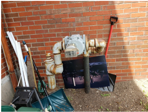
Site Utilities: Central gas meter found at the site.
