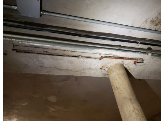
Foundation: Typical cracks on basement walls and ceilings found throughout the site. (Critical Repair)
