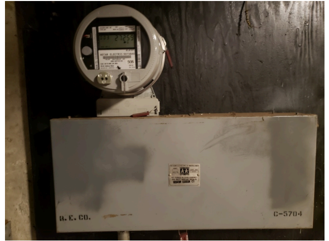
26. Site Utilities: Central electric meter found at the site.
