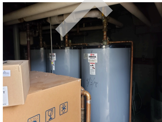
Plumbing: Storage tanks found on the property.
