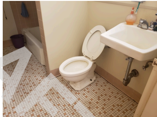
Cabinets & Fixtures: Typical dwelling unit porcelain sink and toilet found throughout the site.
