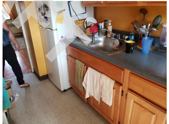
124. Cabinets & Fixtures: Typical dwelling unit kitchen sink, countertop, and wood cabinets found throughout the site.
