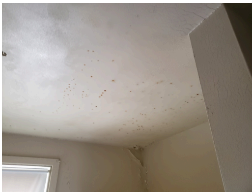
Dwelling Unit Interior Elements: Damaged finishes observed in unit 20. (Non-Critical Repair)
