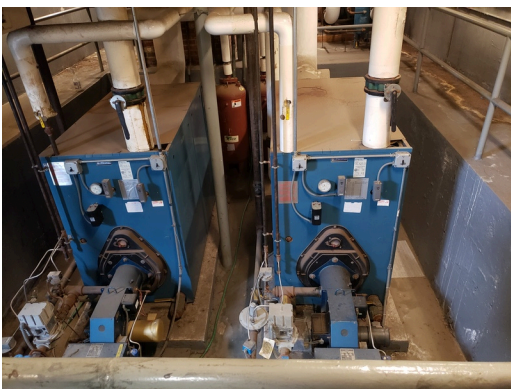
Central gas-fired boilers found on the property.
