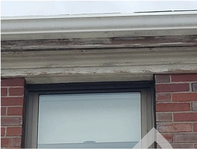
37. Attics & Eaves: Typical perforated eaves vents found throughout the site (Non-Critical Repair)
