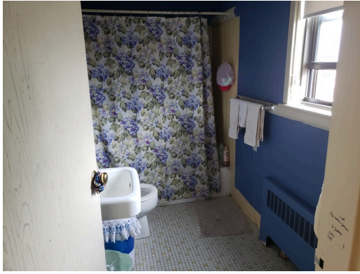
Dwelling Unit Interior Elements: Typical tile flooring and sheetrock finish found in dwelling units throughout the site.
