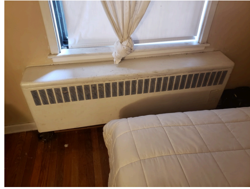
HVAC Systems: Typical hydronic radiant heater found in dwelling units throughout the property.
