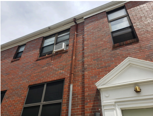
83. HVAC Systems: Typical tenant owned window unit AC system found throughout the site.
