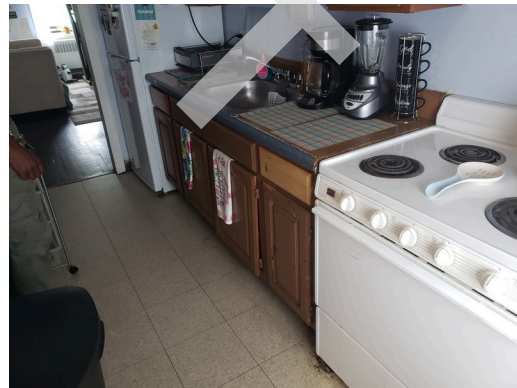
Dwelling Unit Interior Elements: Typical vinyl flooring and sheetrock finish found in dwelling units throughout the site.
