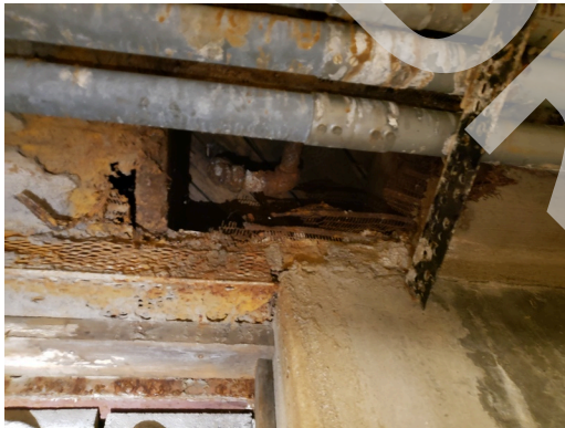
Foundation: Typical cracks on basement walls and ceilings found throughout the site. (Critical Repair)
