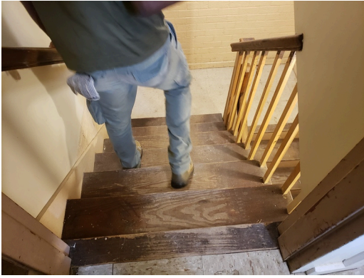
Common Area Interior Elements: Typical staircase with worn down finishes found throughout the site. (Non-Critical Repair)
