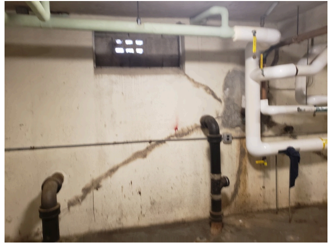
34. Foundation: Typical cracks on basement walls and ceilings found throughout the site. (Critical Repair)
