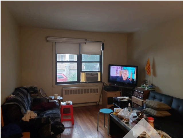
105. Dwelling Unit Interior Elements: Typical wood laminate flooring and sheetrock finish found in dwelling units throughout the site.
