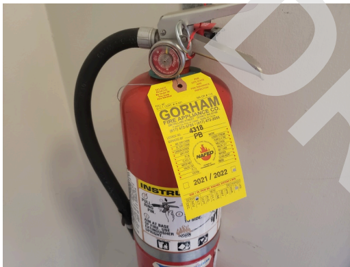
Life & Fire Safety: Typical fire extinguisher found throughout the site.
