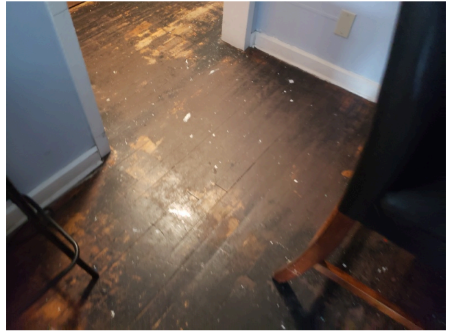
110. Dwelling Unit Interior Elements: Damaged finishes observed in unit 4. (Non-Critical Repair)
