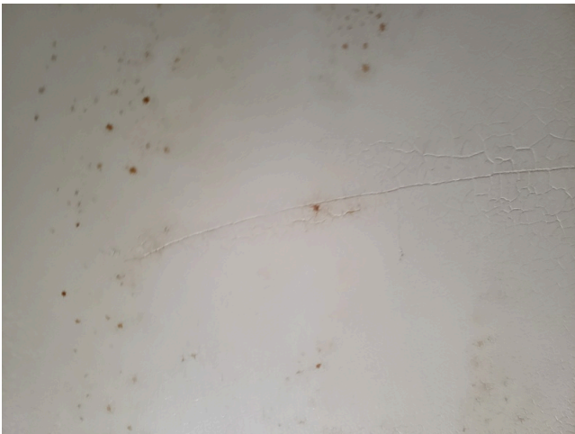
119. Dwelling Unit Interior Elements: Damaged finishes observed in unit 20. (Non-Critical Repair)
