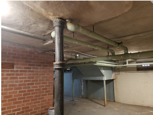
Plumbing: Typical cast iron and PVC waste pipes found throughout the property.
