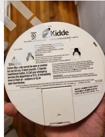
96. Life & Fire Safety: Typical non-compliant smoke detector found throughout the site. (Critical Repair)
