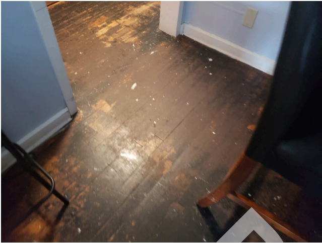
5. Building 1; Unit: 4; Floor: 2; Style: 2 Bed / 1 Bath: Damaged living room finishes. (Non-Critical Repair)
