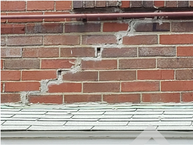
45. Sidewall System: Typical cracked unpainted brick found throughout the site. (Non-Critical Repair)
