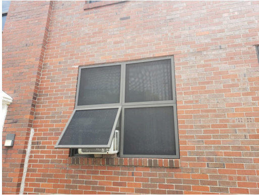
HVAC Systems: Typical tenant owned window unit AC system found throughout the site.
