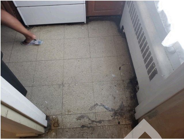
109. Dwelling Unit Interior Elements: Damaged finishes observed in unit 4. (Non-Critical Repair)
