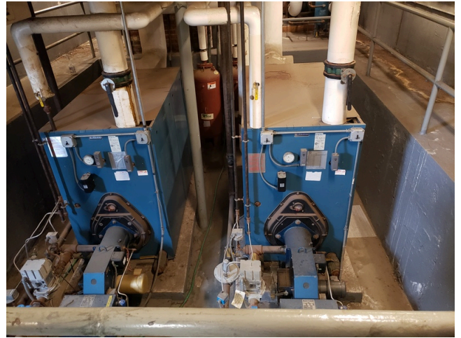
78. Central gas-fired boilers found on the property.
