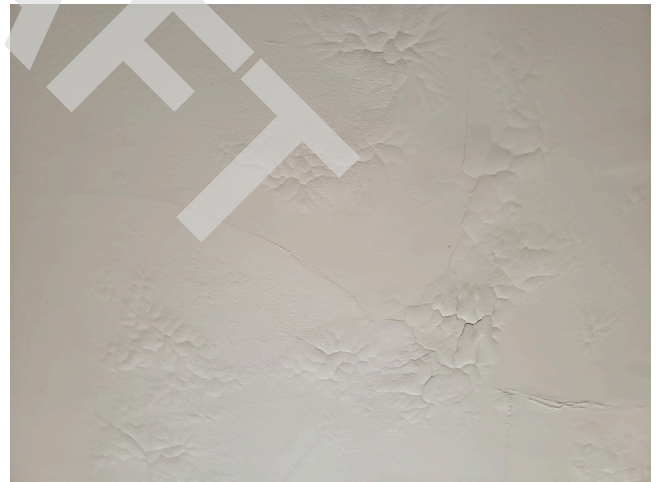
116. Dwelling Unit Interior Elements: Damaged finishes observed in unit 20. (Non-Critical Repair)
