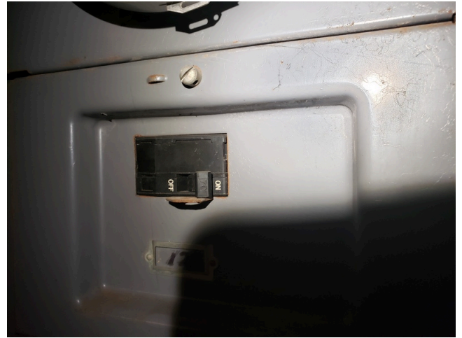
90. Electrical System: Typical master breaker found throughout the site.
