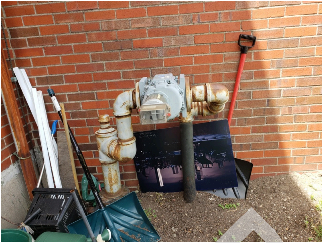
25. Site Utilities: Central gas meter found at the site.
