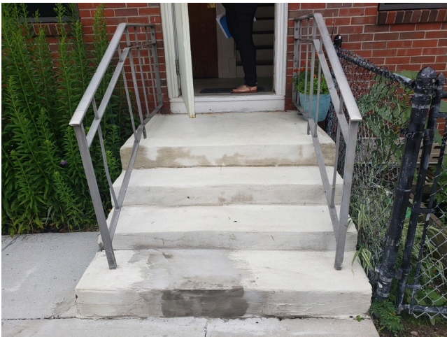
15. Flatwork (Walks, Plazas, Terraces, Patios): Concrete steps with steel handrails found at the property.
