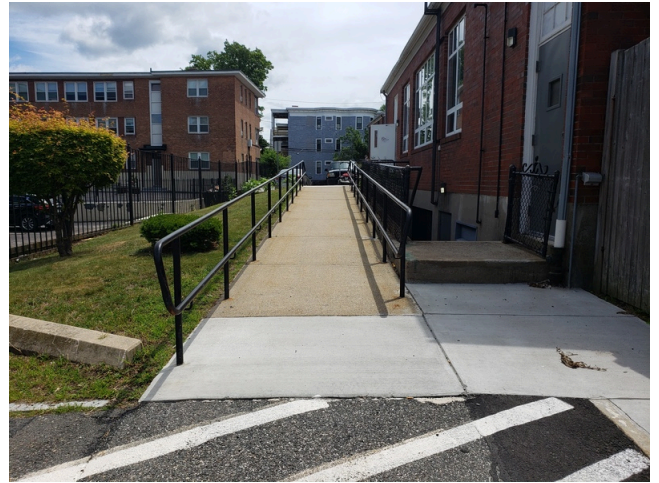
14. Flatwork (Walks, Plazas, Terraces, Patios): Poured in place concrete ramp and sidewalks found at the property.
