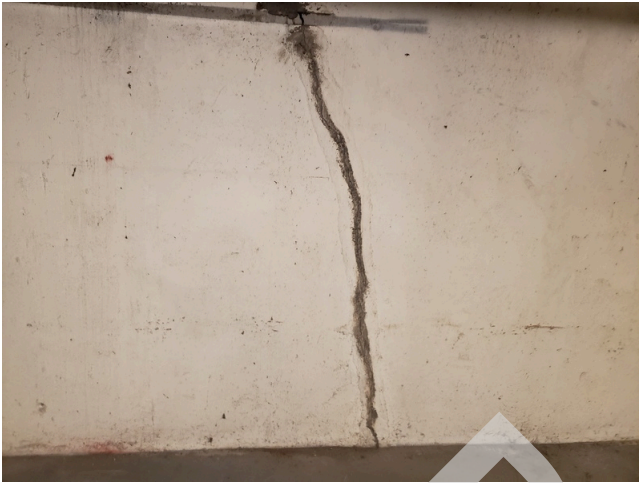
33. Foundation: Typical cracks on basement walls and ceilings found throughout the site. (Critical Repair)
