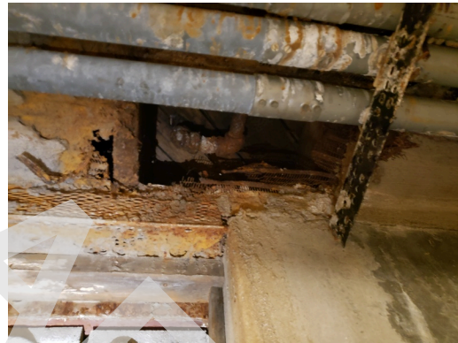
Foundation: Typical cracks on basement walls and ceilings found throughout the site. (Critical Repair)
