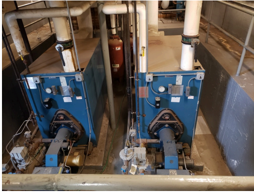
Central gas-fired boilers found on the property.
