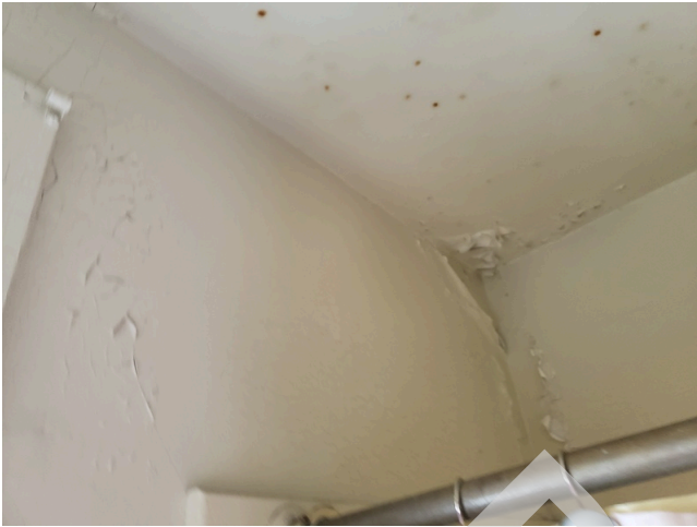
113. Dwelling Unit Interior Elements: Damaged finishes observed in unit 20. (Non-Critical Repair)
