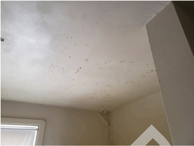
117. Dwelling Unit Interior Elements: Damaged finishes observed in unit 20. (Non-Critical Repair)
