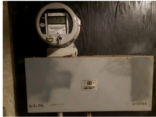
Site Utilities: Central electric meter found at the site.
