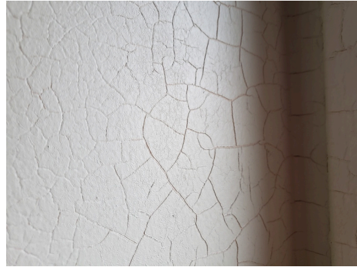
Dwelling Unit Interior Elements: Damaged finishes observed in unit 20. (Non-Critical Repair)
