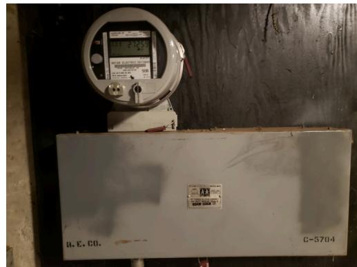
Electrical System: Central electric meter found at the site.
