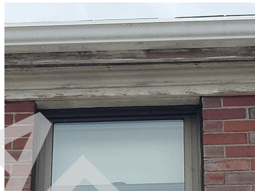
Sidewall System: Typical weathered and damaged wood trim found throughout the site. (Non-Critical Repair)
