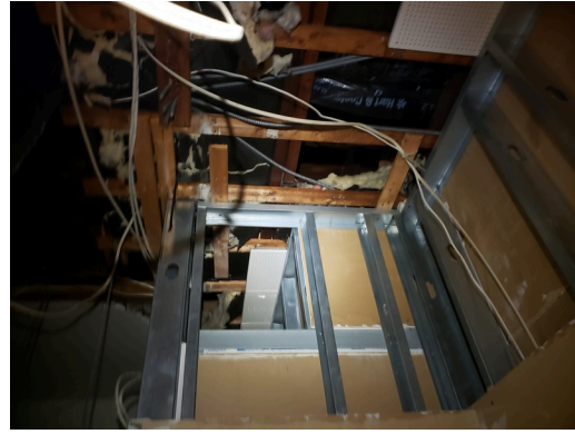
Dwelling Unit Interior Elements: Typical damaged sheetrock ceilings found throughout the site. (Non-Critical Repair)
