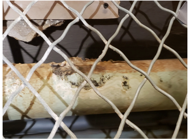
130. Moisture and Microbial Growth: Mold on water pipes observed throughout the site. (Critical Repair)
