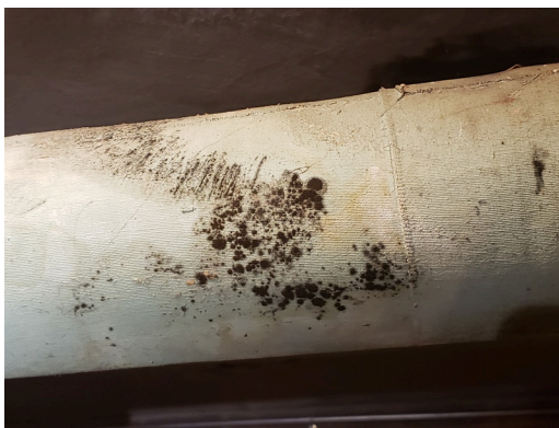
Moisture and Microbial Growth: Mold on water pipes observed throughout the site. (Critical Repair)
