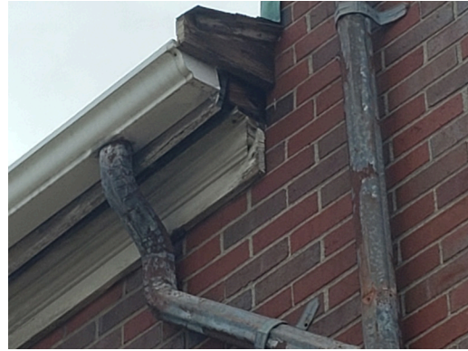
Sidewall System: Typical weathered and damaged wood trim found throughout the site. (Non-Critical Repair)
