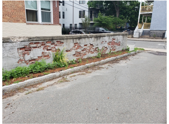
6. Landscaping & Appurtenances: Damaged CMU wall found on the north perimeter of the property. (Non-Critical Repair)
