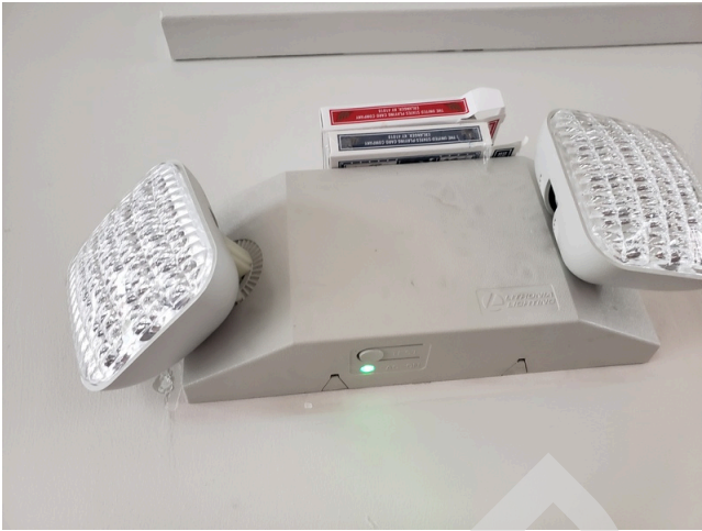
93. Life & Fire Safety: Typical emergency lighting found throughout the site.
