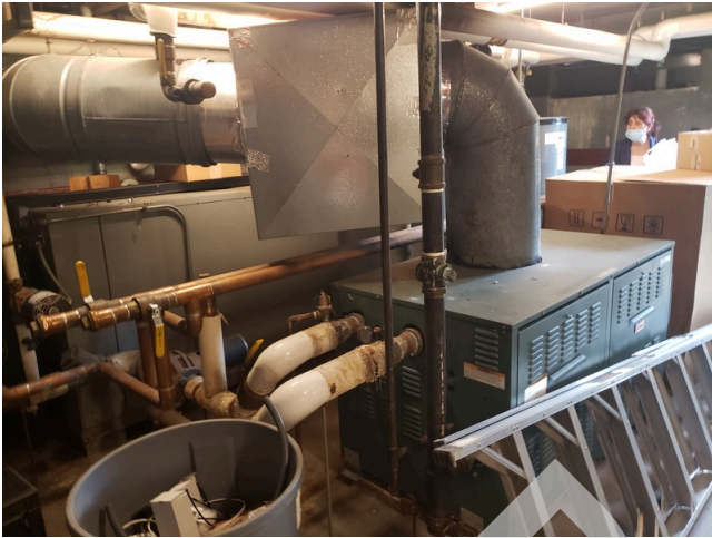
85. Central gas boilers found on the property.
