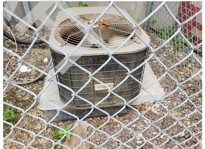
84. HVAC Systems: 3 ton AC system found at the community room.
