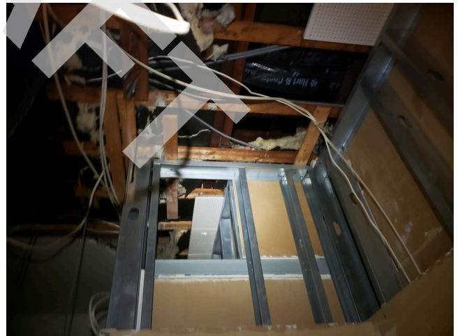
120. Dwelling Unit Interior Elements: Typical damaged sheetrock ceilings found throughout the site. (Non-Critical Repair)
