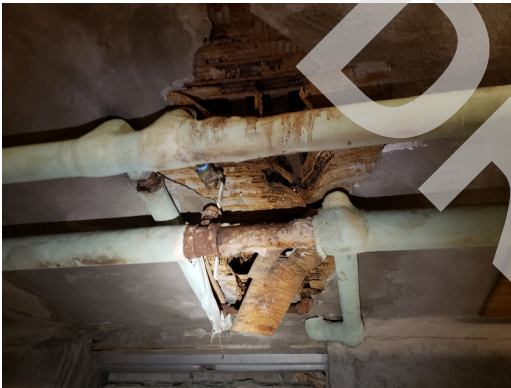
Foundation: Typical cracks on basement walls and ceilings found throughout the site. (Critical Repair)
