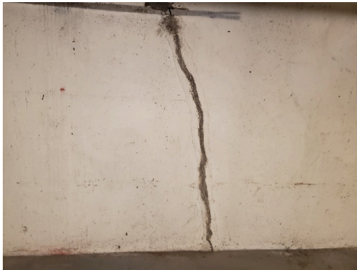
Foundation: Typical cracks on basement walls and ceilings found throughout the site. (Critical Repair)
