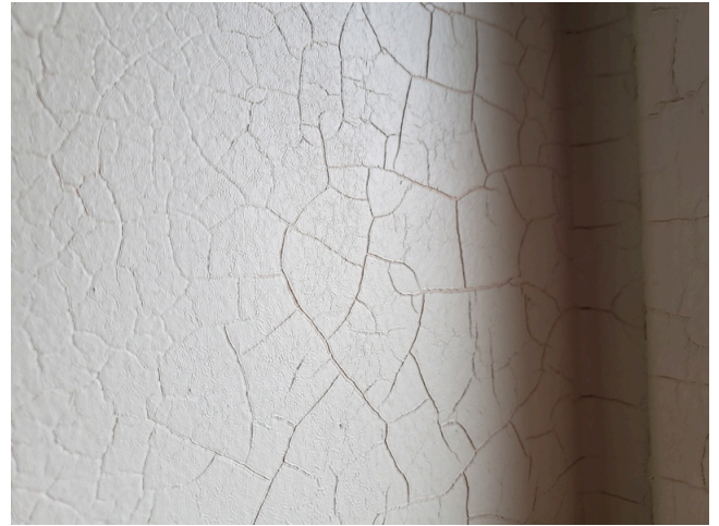
114. Dwelling Unit Interior Elements: Damaged finishes observed in unit 20. (Non-Critical Repair)
