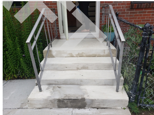
Flatwork (Walks, Plazas, Terraces, Patios): Concrete steps with steel handrails found at the property.
