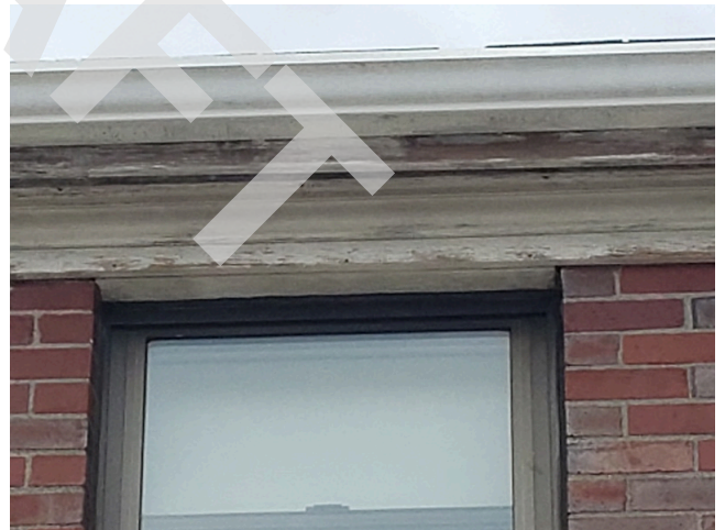
48. Sidewall System: Typical weathered and damaged wood trim found throughout the site. (Non-Critical Repair)
