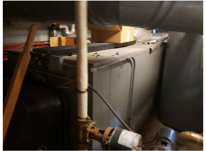
86. Central gas boilers found on the property.
