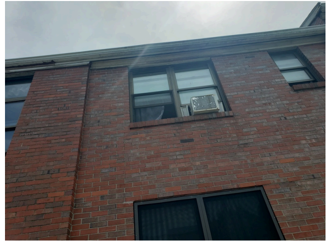
82. HVAC Systems: Typical tenant owned window unit AC system found throughout the site.
