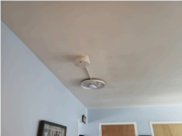
95. Life & Fire Safety: Typical non-compliant smoke detector found throughout the site. (Critical Repair)
