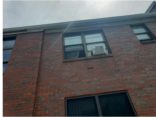
HVAC Systems: Typical tenant owned window unit AC system found throughout the site.
