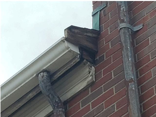
47. Sidewall System: Typical weathered and damaged wood trim found throughout the site. (Non-Critical Repair)
