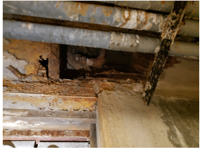
30. Foundation: Typical cracks on basement walls and ceilings found throughout the site. (Critical Repair)
