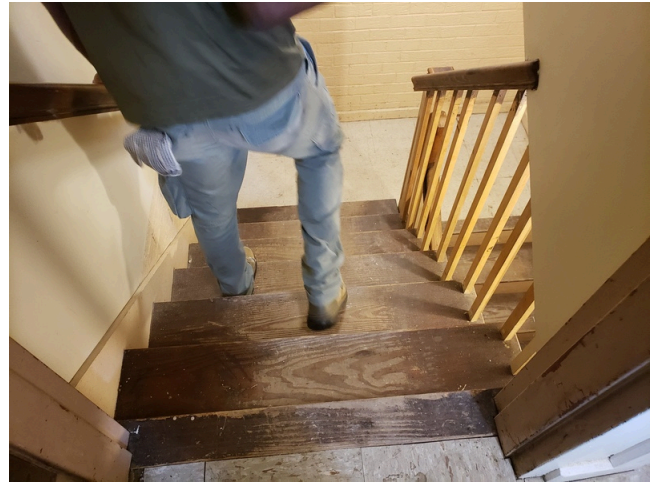
102. Common Area Interior Elements: Typical staircase with worn down finishes found throughout the site. (Non-Critical Repair)
