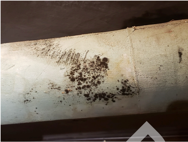
129. Moisture and Microbial Growth: Mold on water pipes observed throughout the site. (Critical Repair)
