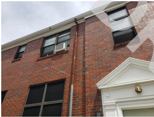
HVAC Systems: Typical tenant owned window unit AC system found throughout the site.
