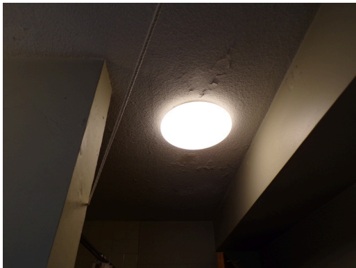
Bathroom Light Fixture
