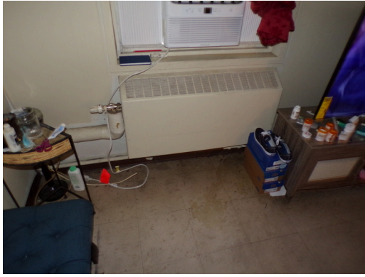
Dwelling unit radiator
