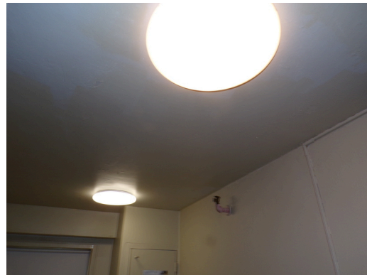
Kitchen Light Fixtures
