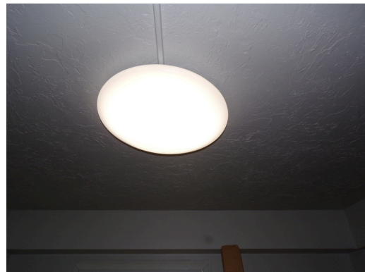
Storage Room Lighting
