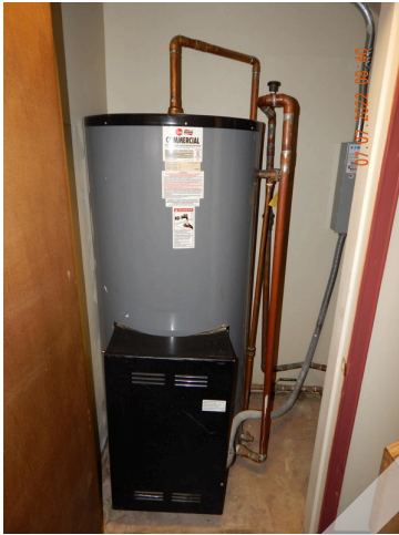
113. Plumbing: Typical central electric water heater found at the property.
