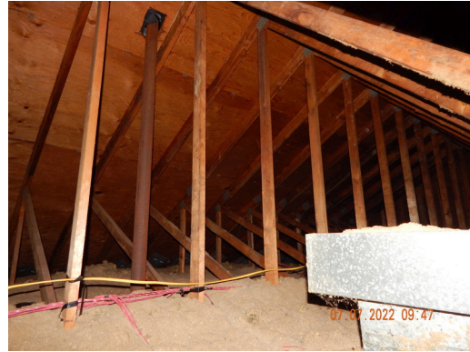
Insulation: Typical blown-in cellulose and fiber glass batt insulation found throughout the site.
