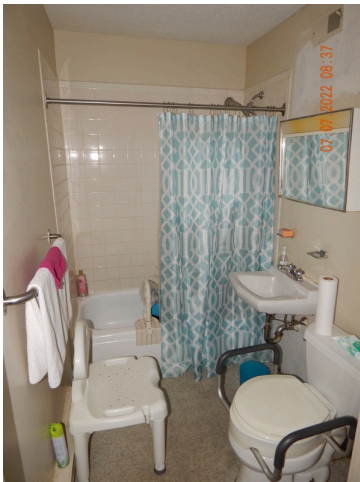
155. Cabinets & Fixtures: Typical dwelling unit enamel tub and tile surround found throughout the site.
