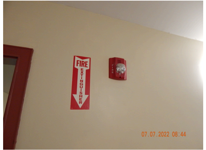
130. Life & Fire Safety: Typical strobe light found in common areas throughout the site.
