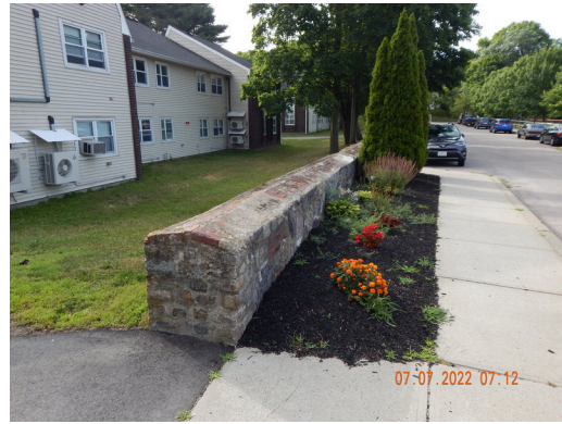
Landscaping & Appurtenances: Damaged Masonry wall found on the south perimeter of the property. (Non-Critical Repair)
