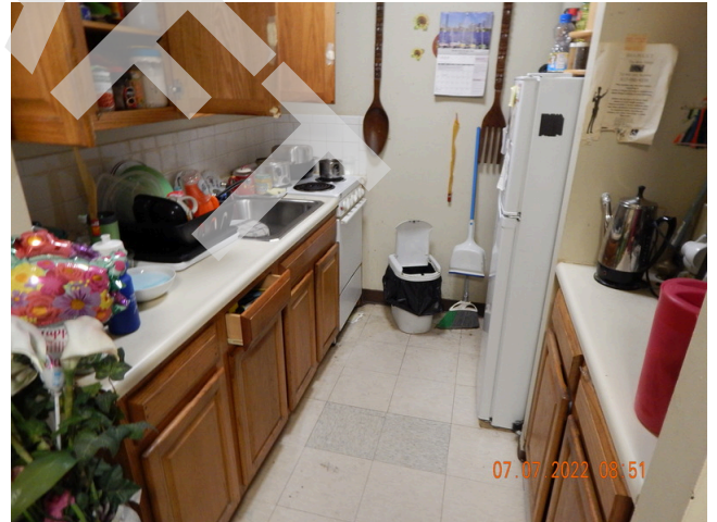
144. Dwelling Unit Interior Elements: Typical vinyl flooring and sheetrock finish found in dwelling units throughout the site.
