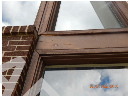
Sidewall System: Typical damaged or weathered wood trim found throughout the community building. (Non-Critical Repair)
