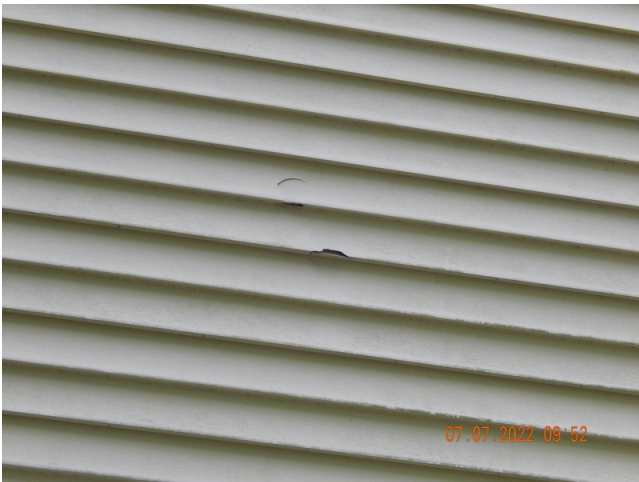
71. Sidewall System: Typical damaged or weathered sidewall vinyl siding found throughout the site. (Non-Critical Repair)
