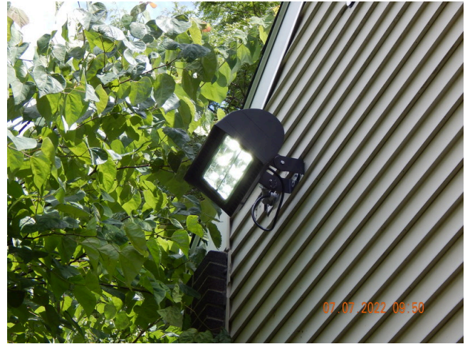
30. Landscaping & Appurtenances: Typical building lighting found throughout the property.
