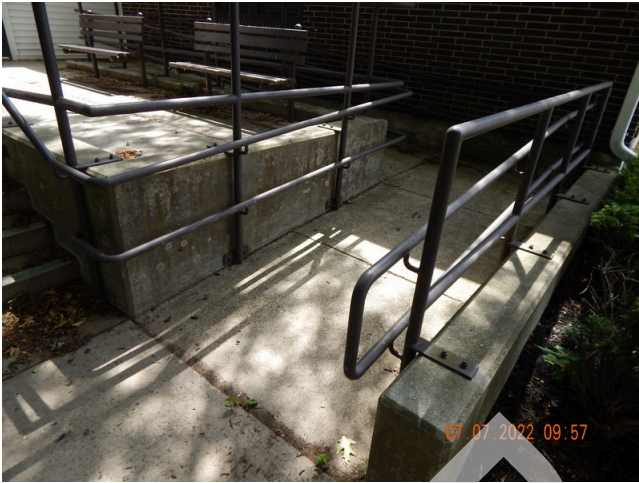
21. Flatwork (Walks, Plazas, Terraces, Patios): Poured in place concrete ramp found at the property.
