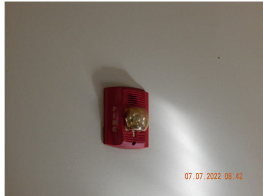
Life & Fire Safety: Typical strobe light found in individual units throughout the site.
