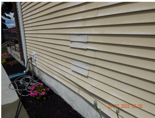
Sidewall System: Typical damaged or weathered sidewall vinyl siding found throughout the site. (Non-Critical Repair)
