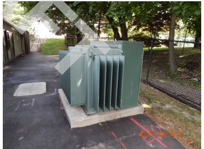
36. Site Utilities: Typical pad-mounted transformer found at the site.
