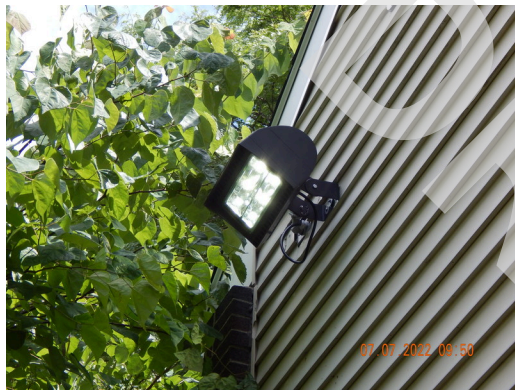
Landscaping & Appurtenances: Typical building lighting found throughout the property.
