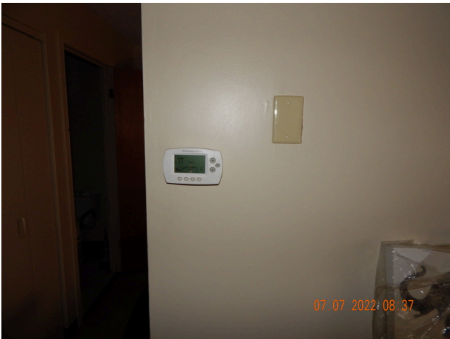
123. HVAC Systems: Typical thermostat found throughout the site.
