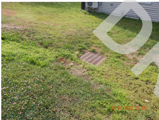
Stormwater Drainage: Typical landscaping drainage found throughout site.
