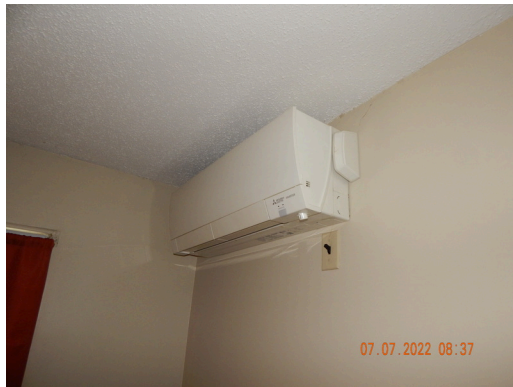
HVAC Systems: Typical individual heat pump units found throughout the site.
