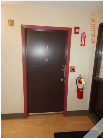
57. Exterior Doors & Entry Systems: Typical metal-clad unit door found throughout the site.
