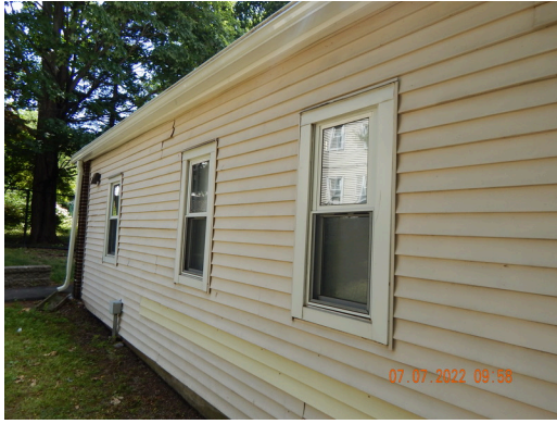
Sidewall System: Typical damaged or weathered sidewall vinyl siding found throughout the site. (Non-Critical Repair)
