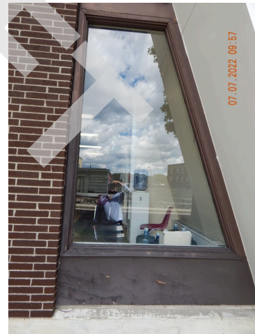
76. Sidewall System: Typical damaged or weathered wood trim found throughout the community building. (Non-Critical Repair)
