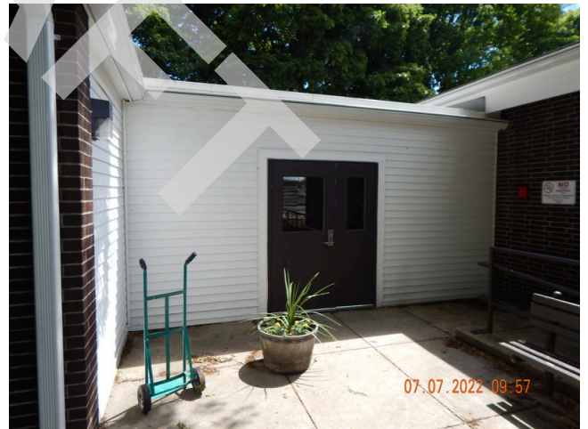
60. Exterior Doors & Entry Systems: Typical community building access door found throughout the site.
