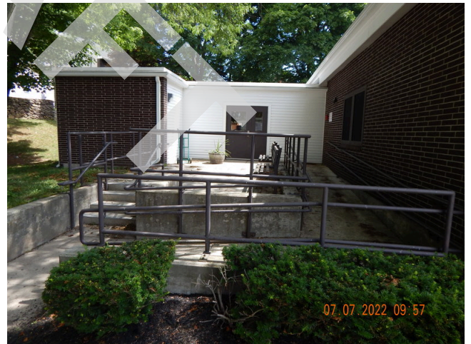
20. Flatwork (Walks, Plazas, Terraces, Patios): Poured in place concrete ramp and sidewalks found at the property.
