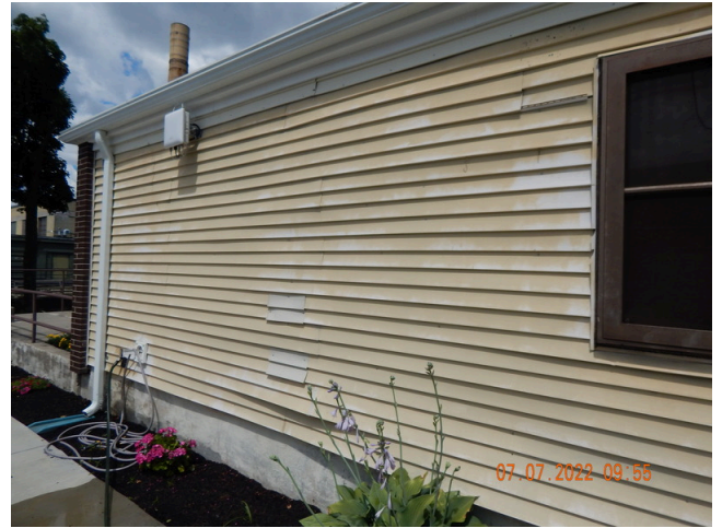
66. Sidewall System: Typical damaged or weathered sidewall vinyl siding found throughout the site. (Non-Critical Repair)
