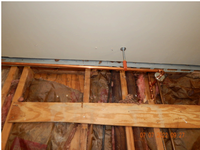
115. Plumbing: Typical copper distribution pipes found throughout property.
