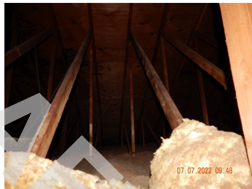
Roof Frame & Sheathing: Typical wood trusses and plywood decking found throughout the property.
