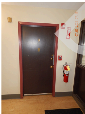
Exterior Doors & Entry Systems: Typical metal-clad unit door found throughout the site.
