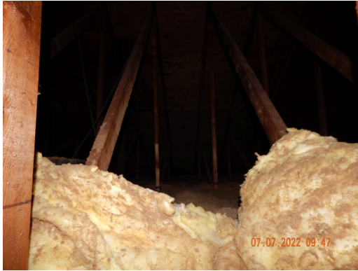
Insulation: Typical blown-in cellulose and fiber glass batt insulation found throughout the site.
