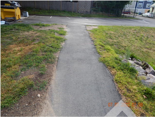
17. Flatwork (Walks, Plazas, Terraces, Patios): Typical asphalt sidewalk found around the property.
