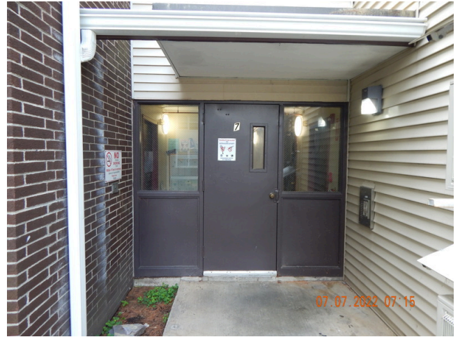
58. Exterior Doors & Entry Systems: Typical building access door found throughout the site.
