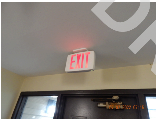
Life & Fire Safety: Typical illuminated exit sign found throughout the site.
