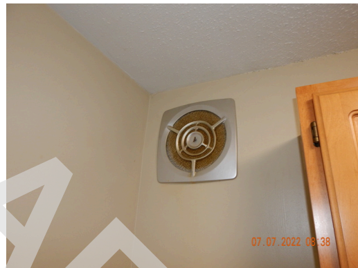
HVAC Systems: Typical kitchen exhaust fan found throughout the site.
