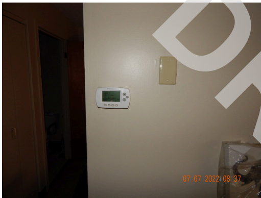
HVAC Systems: Typical thermostat found throughout the site.
