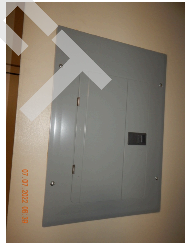
128. Electrical System: Typical dwelling unit electric panel found throughout the site.
