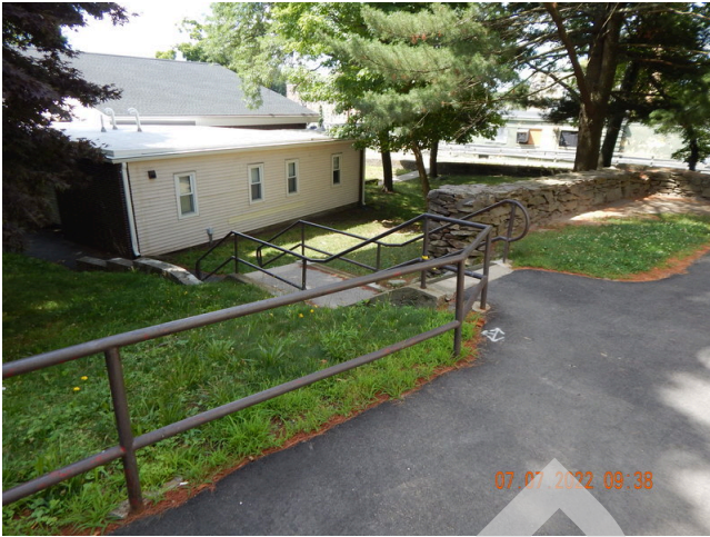
25. Flatwork (Walks, Plazas, Terraces, Patios): Typical steel handrails found at the property.
