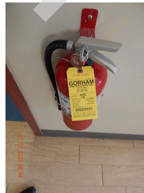
Life & Fire Safety: Typical fire extinguisher found throughout the site.
