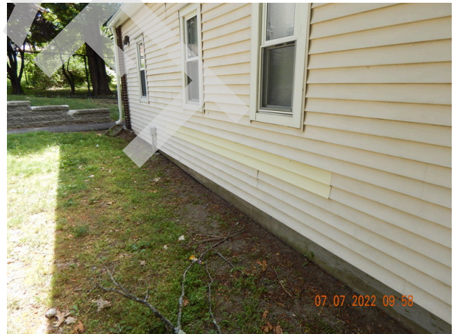
68. Sidewall System: Typical damaged or weathered sidewall vinyl siding found throughout the site. (Non-Critical Repair)
