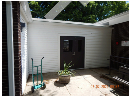
Exterior Doors & Entry Systems: Typical community building access door found throughout the site.
