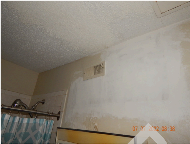
125. HVAC Systems: Typical bathroom exhaust fan found throughout the site.
