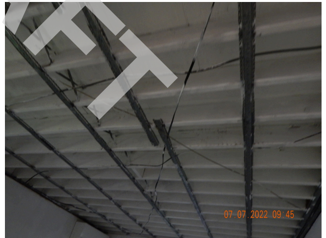
148. Dwelling Unit Interior Elements: Unit 42 gutted and unfinished. (Critical Repair)
