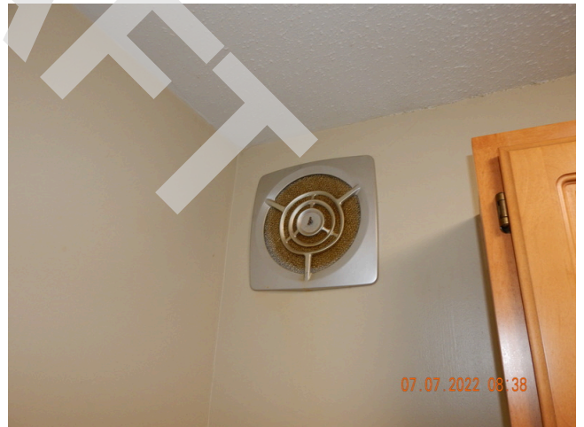
124. HVAC Systems: Typical kitchen exhaust fan found throughout the site.
