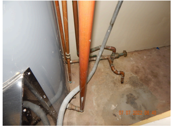
114. Plumbing: Typical copper distribution pipes found throughout property.
