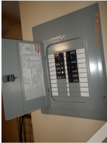
129. Electrical System: Typical dwelling unit electric panel found throughout the site.
