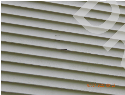
Sidewall System: Typical damaged or weathered sidewall vinyl siding found throughout the site. (Non-Critical Repair)
