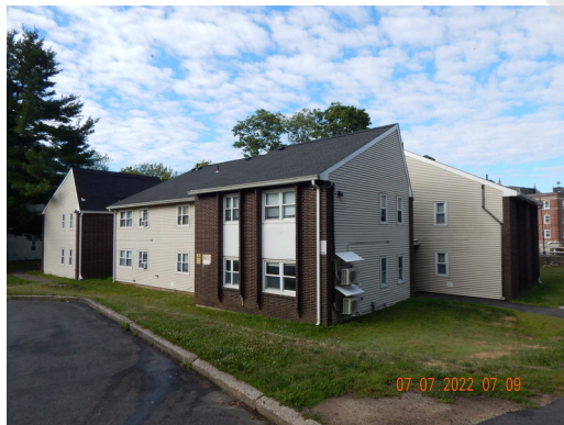
Sidewall System: Typical sidewall vinyl siding and unpainted brick found throughout the site.
