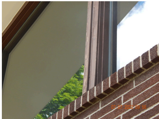
Sidewall System: Typical damaged or weathered wood trim found throughout the community building. (Non-Critical Repair)
