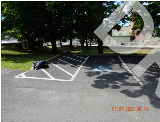
Paving, Curbing, & Parking: Typical accessible parking spaces found throughout the property, missing vertical sign (Critical Repair)
