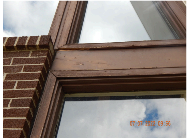
78. Sidewall System: Typical damaged or weathered wood trim found throughout the community building. (Non-Critical Repair)
