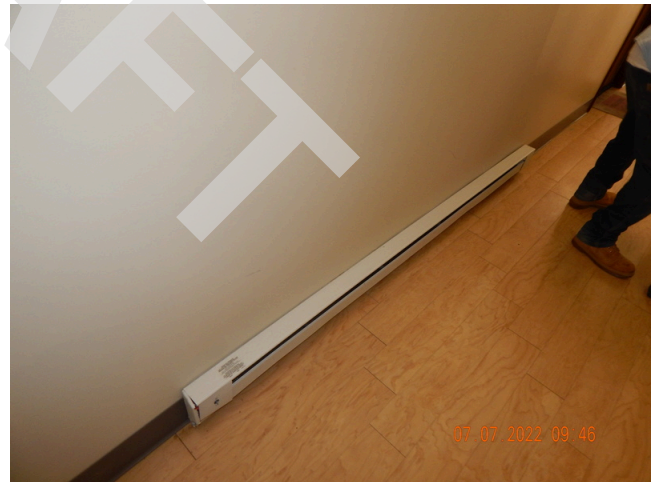
120. HVAC Systems: Typical electric baseboard heater found in common areas throughout the site.
