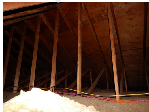
Roof Frame & Sheathing: Typical wood trusses and plywood decking found throughout the property.
