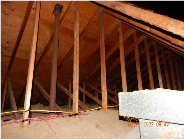
45. Roof Frame & Sheathing: Typical wood trusses and plywood decking found throughout the property.
