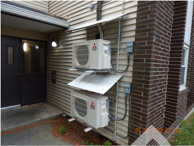
117. HVAC Systems: Typical 1.5 ton individual heat pump units found throughout the site.
