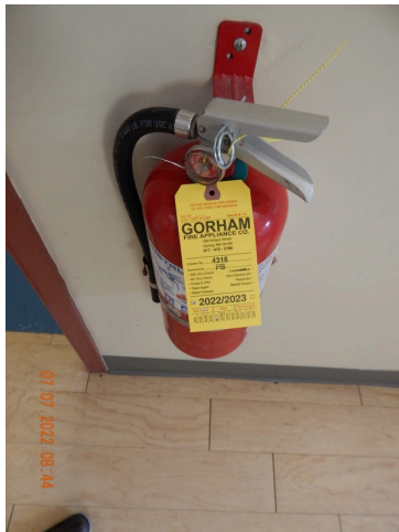
135. Life & Fire Safety: Typical fire extinguisher found throughout the site.
