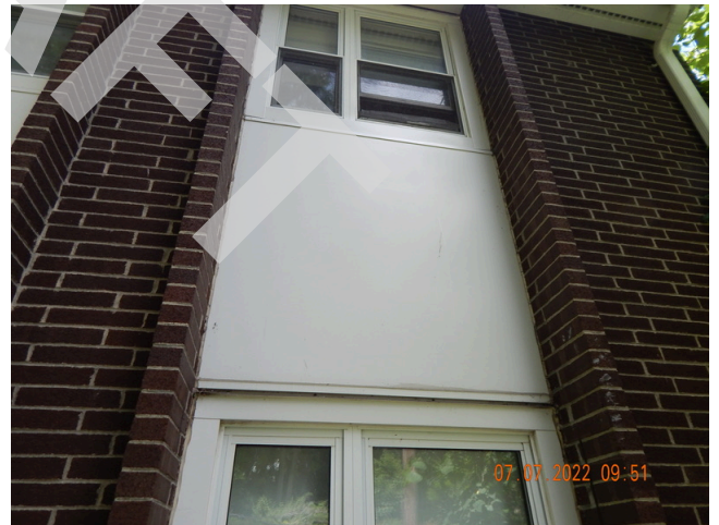
40. Framing System, Floors & Walls: Typical steel lintels at window and door openings found throughout the site.
