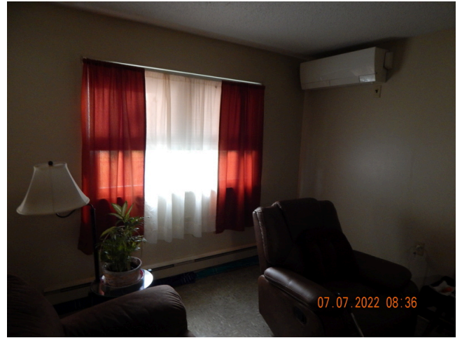
142. Dwelling Unit Interior Elements: Typical vinyl flooring and sheetrock finish found in dwelling units throughout the site.
