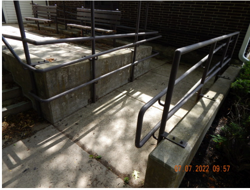
Flatwork (Walks, Plazas, Terraces, Patios): Poured in place concrete ramp found at the property.
