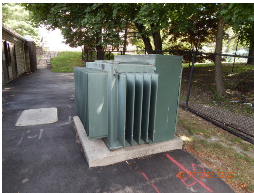
Site Utilities: Typical pad-mounted transformer found at the site.
