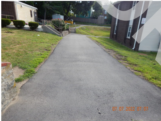
Flatwork (Walks, Plazas, Terraces, Patios): Typical asphalt sidewalk found around the property.
