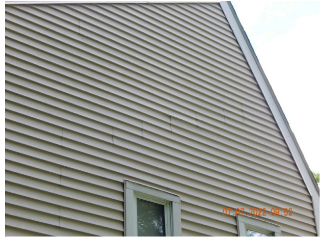
70. Sidewall System: Typical damaged or weathered sidewall vinyl siding found throughout the site. (Non-Critical Repair)
