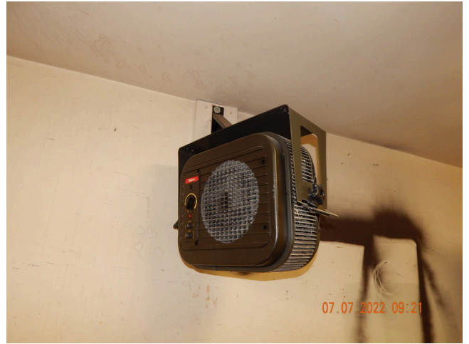
122. HVAC Systems: Typical electric ceiling mounted heater found in common areas throughout the site.
