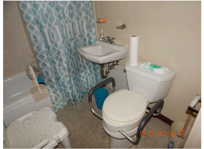
154. Cabinets & Fixtures: Typical dwelling unit porcelain sink and toilet found throughout the site.
