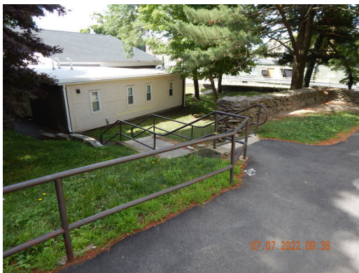
Flatwork (Walks, Plazas, Terraces, Patios): Typical steel handrails found at the property.
