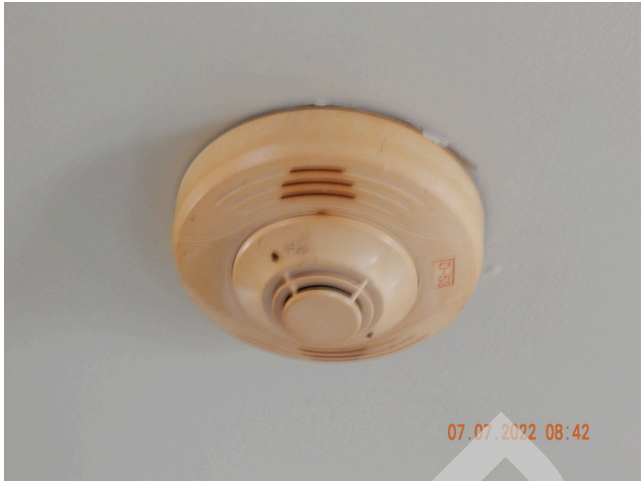
133. Life & Fire Safety: Typical hardwired smoke detector found throughout the site.
