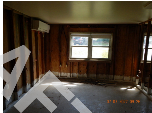
Dwelling Unit Interior Elements: Unit 26 gutted and unfinished. (Critical Repair)
