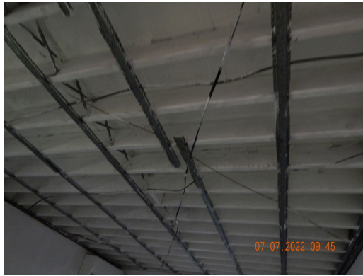
Dwelling Unit Interior Elements: Unit 42 gutted and unfinished. (Critical Repair)
