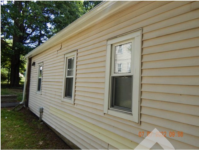
69. Sidewall System: Typical damaged or weathered sidewall vinyl siding found throughout the site. (Non-Critical Repair)
