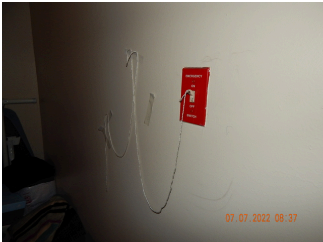
7. Building 1; Unit: 1F; Floor: 1; Style: Studio: Emergency pull cord.
