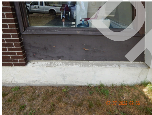
Sidewall System: Typical damaged or weathered wood trim found throughout the community building. (Non-Critical Repair)
