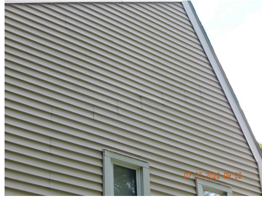
Sidewall System: Typical damaged or weathered sidewall vinyl siding found throughout the site. (Non-Critical Repair)
