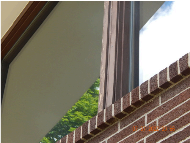
79. Sidewall System: Typical damaged or weathered wood trim found throughout the community building. (Non-Critical Repair)
