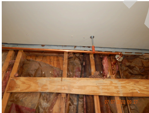
Plumbing: Typical copper distribution pipes found throughout property.
