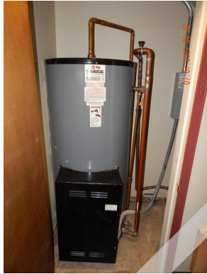
Plumbing: Typical central electric water heater found at the property.
