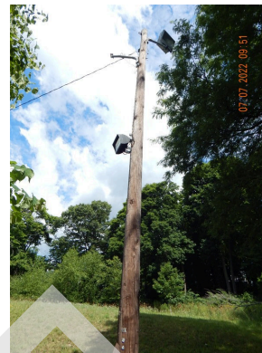
Landscaping & Appurtenances: Typical parking area lighting found throughout the property.
