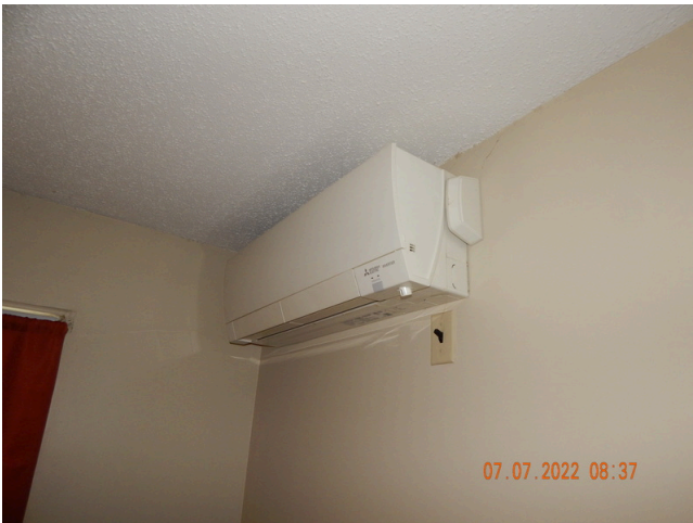
119. HVAC Systems: Typical individual heat pump units found throughout the site.
