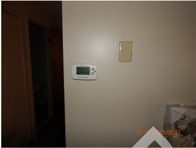
5. Building 1; Unit: 1F; Floor: 1; Style: Studio: Thermostat.
