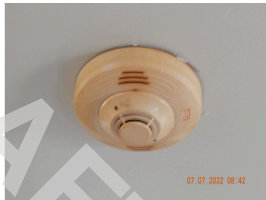
Life & Fire Safety: Typical hardwired smoke detector found throughout the site.
