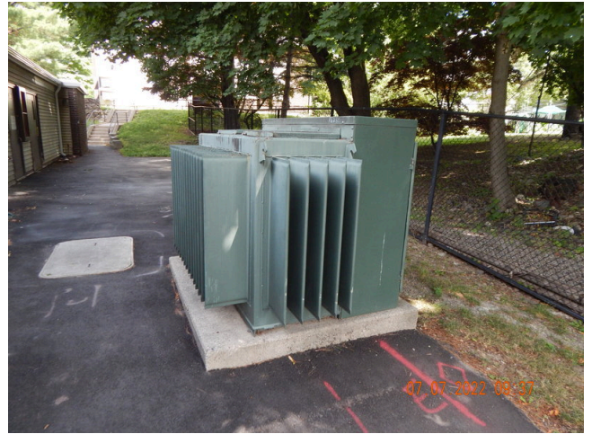
126. Electrical System: Typical pad-mounted transformer found at the site.
