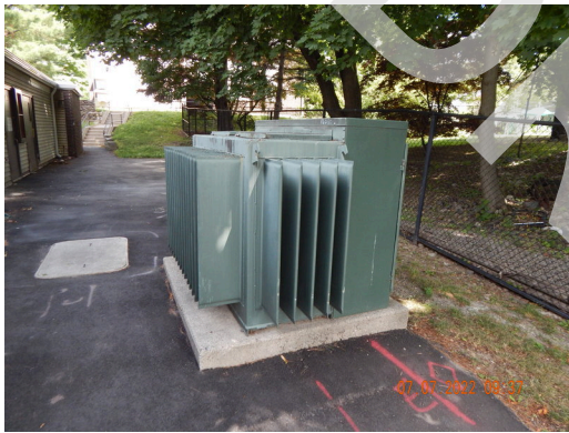
Electrical System: Typical pad-mounted transformer found at the site.
