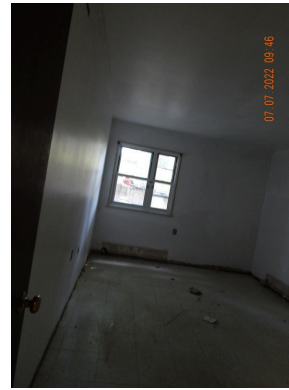
Dwelling Unit Interior Elements: Unit 42 gutted and unfinished. (Critical Repair)
