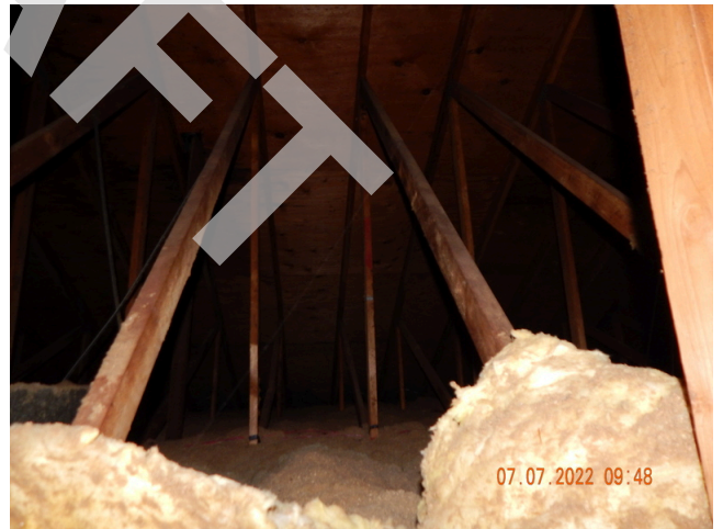
56. Insulation: Typical blown-in cellulose and fiber glass batt insulation found throughout the site.
