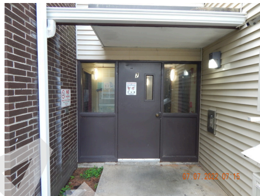
Exterior Doors & Entry Systems: Typical building access door found throughout the site.
