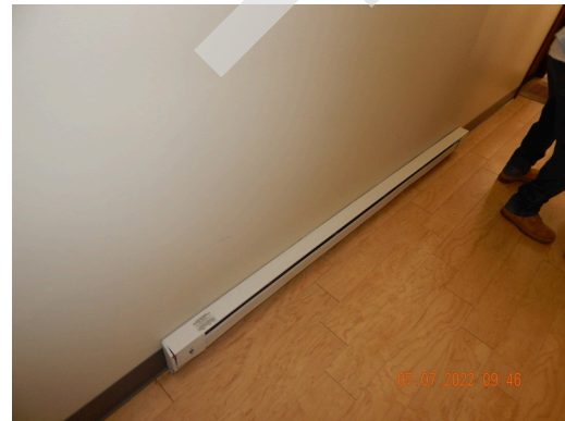
HVAC Systems: Typical electric baseboard heater found in common areas throughout the site.
