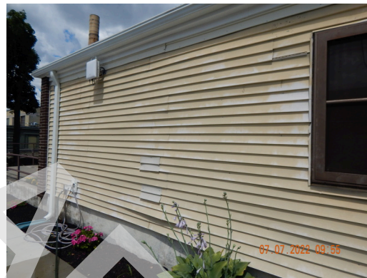
Sidewall System: Typical damaged or weathered sidewall vinyl siding found throughout the site. (Non-Critical Repair)
