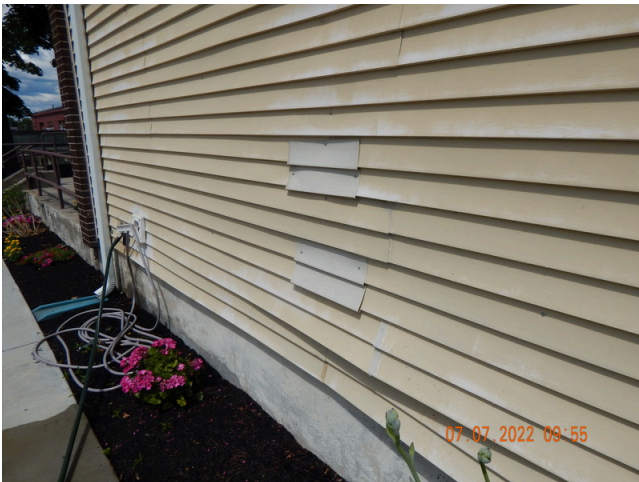
67. Sidewall System: Typical damaged or weathered sidewall vinyl siding found throughout the site. (Non-Critical Repair)
