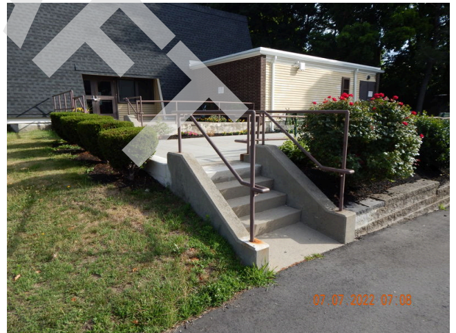
24. Flatwork (Walks, Plazas, Terraces, Patios): Concrete steps with steel handrails found at the property.
