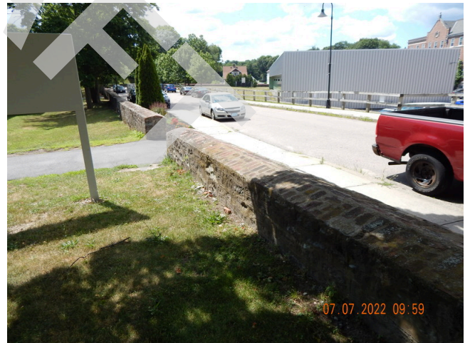
28. Landscaping & Appurtenances: Damaged Masonry wall found on the south perimeter of the property. (Non-Critical Repair)
