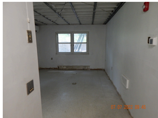
Dwelling Unit Interior Elements: Unit 42 gutted and unfinished. (Critical Repair)
