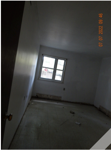
149. Dwelling Unit Interior Elements: Unit 42 gutted and unfinished. (Critical Repair)
