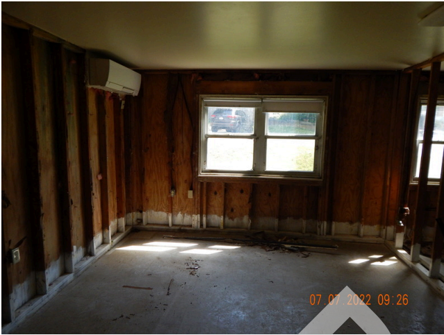
145. Dwelling Unit Interior Elements: Unit 26 gutted and unfinished. (Critical Repair)
