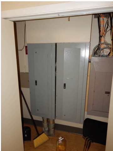
127. Electrical System: Typical central electric panel found throughout the site.
