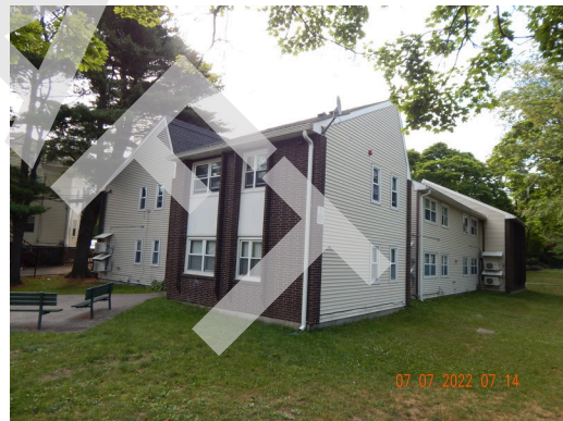
Sidewall System: Typical sidewall vinyl siding and unpainted brick found throughout the site.
