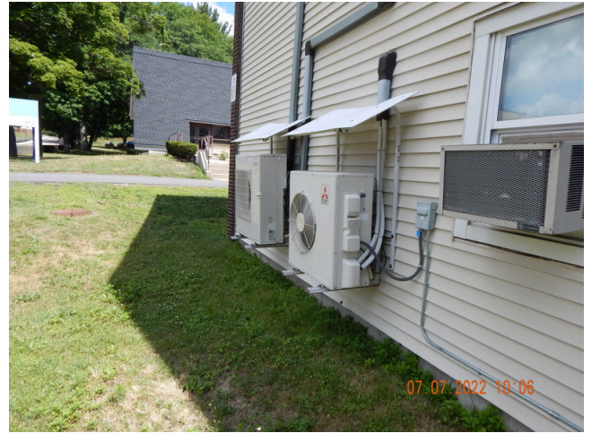
118. HVAC Systems: Typical 2 ton individual heat pump units found throughout the site.
