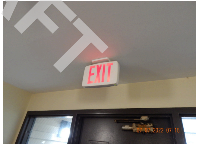
132. Life & Fire Safety: Typical illuminated exit sign found throughout the site.
