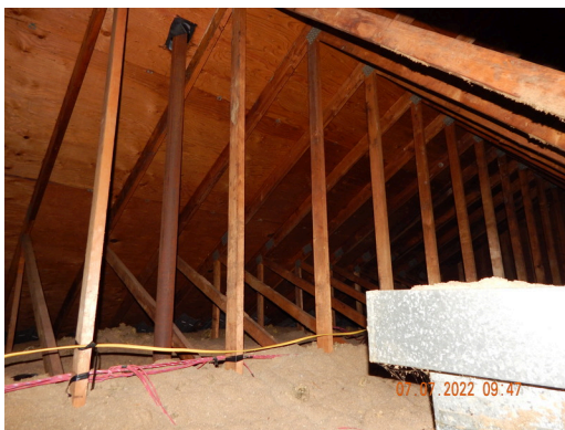
Roof Frame & Sheathing: Typical wood trusses and plywood decking found throughout the property.
