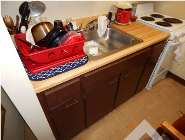
153. Cabinets & Fixtures: Typical dwelling unit kitchen sink, countertop, and wood cabinets found throughout the site.
