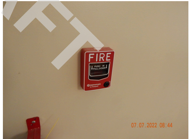
136. Life & Fire Safety: Typical fire alarm system pull found throughout the site.
