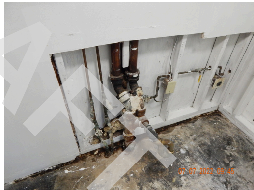
Plumbing: Typical cast iron waste pipes found throughout the property.
