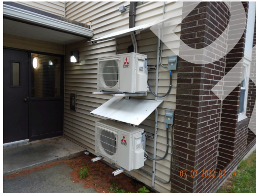
HVAC Systems: Typical 1.5 ton individual heat pump units found throughout the site.
