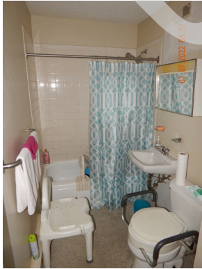
Cabinets & Fixtures: Typical dwelling unit enamel tub and tile surround found throughout the site.
