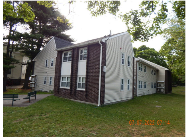
62. Sidewall System: Typical sidewall vinyl siding and unpainted brick found throughout the site.
