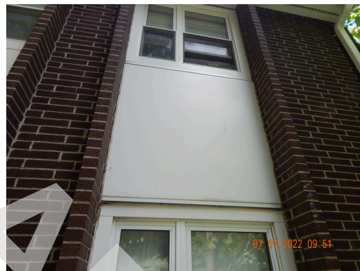
Framing System, Floors & Walls: Typical steel lintels at window and door openings found throughout the site.
