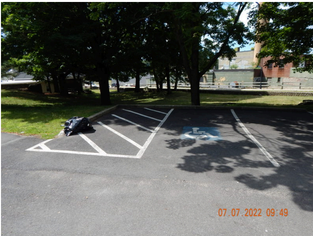
15. Paving, Curbing, & Parking: Typical accessible parking spaces found throughout the property, missing vertical sign (Critical Repair)
