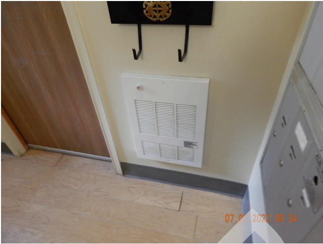
121. HVAC Systems: Typical electric in-wall heater found in common areas throughout the site.
