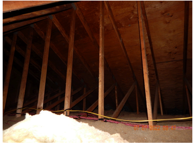
46. Roof Frame & Sheathing: Typical wood trusses and plywood decking found throughout the property.
