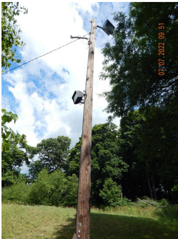
31. Landscaping & Appurtenances: Typical parking area lighting found throughout the property.
