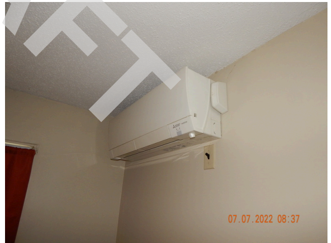
4. Building 1; Unit: 1F; Floor: 1; Style: Studio: Heat pump.
