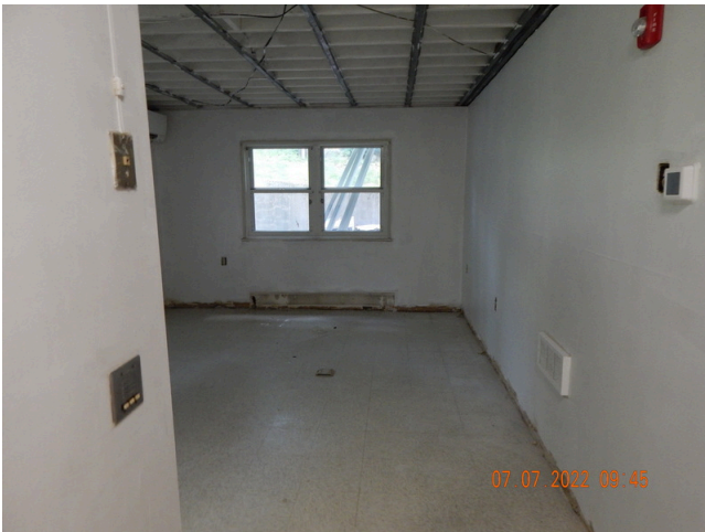
147. Dwelling Unit Interior Elements: Unit 42 gutted and unfinished. (Critical Repair)
