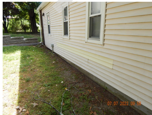
Sidewall System: Typical damaged or weathered sidewall vinyl siding found throughout the site. (Non-Critical Repair)
