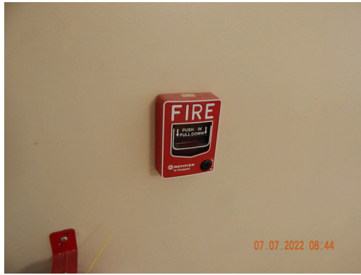
Life & Fire Safety: Typical fire alarm system pull found throughout the site.
