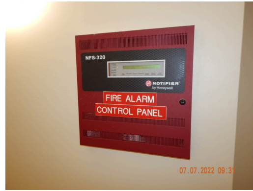
Life & Fire Safety: Fire alarm system found throughout the site (Missing inspection tag). (Critical Repair)
