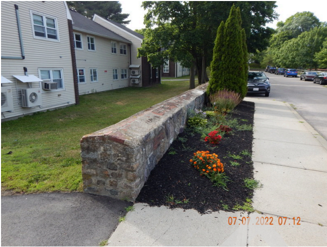
29. Landscaping & Appurtenances: Damaged Masonry wall found on the south perimeter of the property. (Non-Critical Repair)
