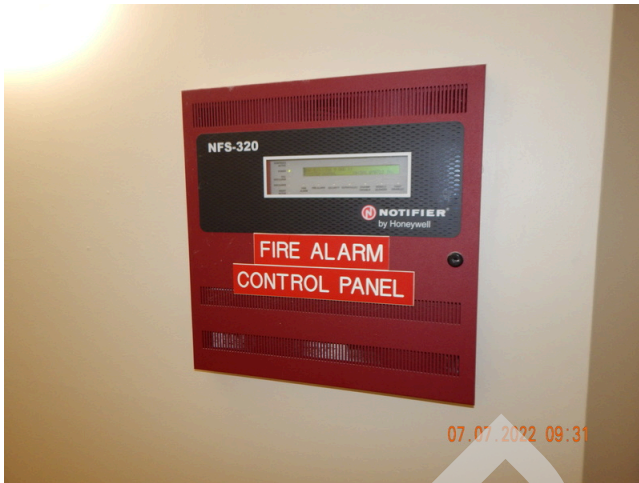
137. Life & Fire Safety: Fire alarm system found throughout the site (Missing inspection tag). (Critical Repair)
