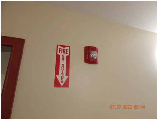
Life & Fire Safety: Typical strobe light found in common areas throughout the site.
