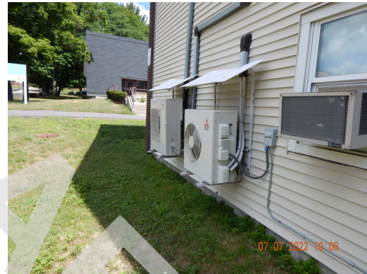
HVAC Systems: Typical 2 ton individual heat pump units found throughout the site.
