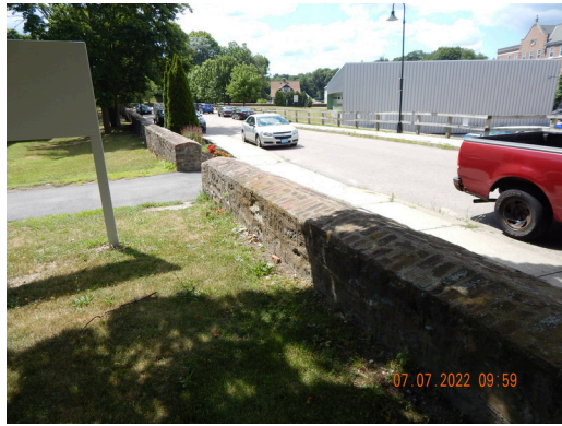
Landscaping & Appurtenances: Damaged Masonry wall found on the south perimeter of the property. (Non-Critical Repair)
