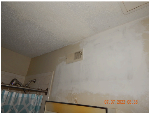
HVAC Systems: Typical bathroom exhaust fan found throughout the site.
