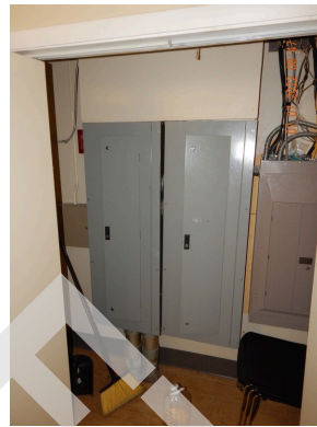
Electrical System: Typical central electric panel found throughout the site.
