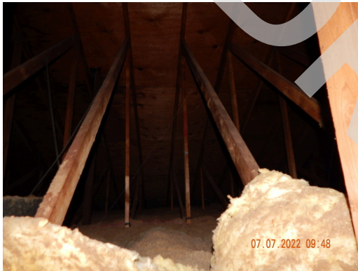
Insulation: Typical blown-in cellulose and fiber glass batt insulation found throughout the site.
