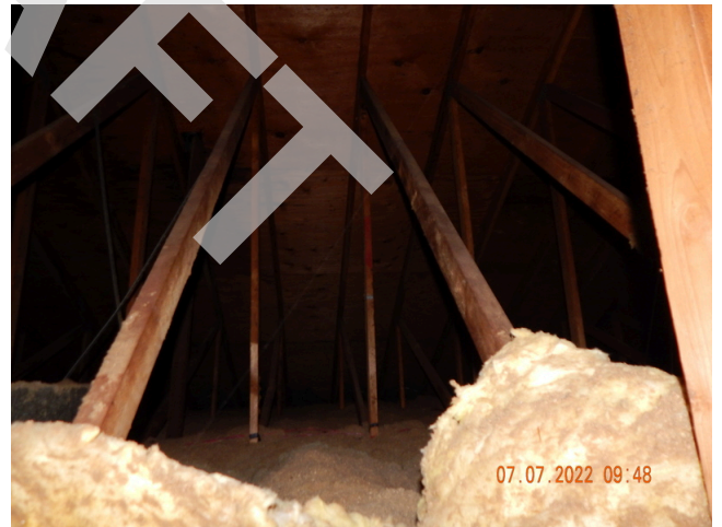
44. Roof Frame & Sheathing: Typical wood trusses and plywood decking found throughout the property.
