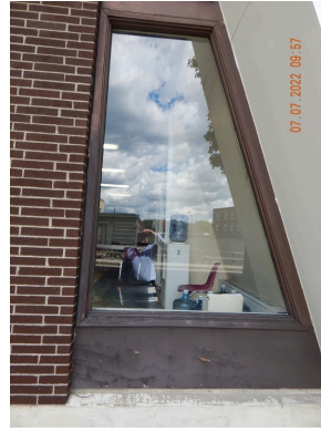
Sidewall System: Typical damaged or weathered wood trim found throughout the community building. (Non-Critical Repair)
