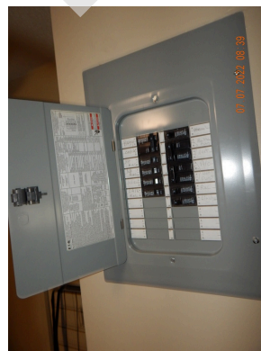
Electrical System: Typical dwelling unit electric panel found throughout the site.
