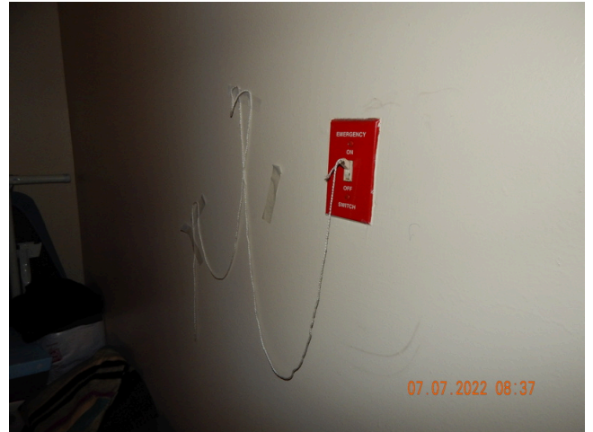
134. Life & Fire Safety: Typical emergency pull cord throughout the site.
