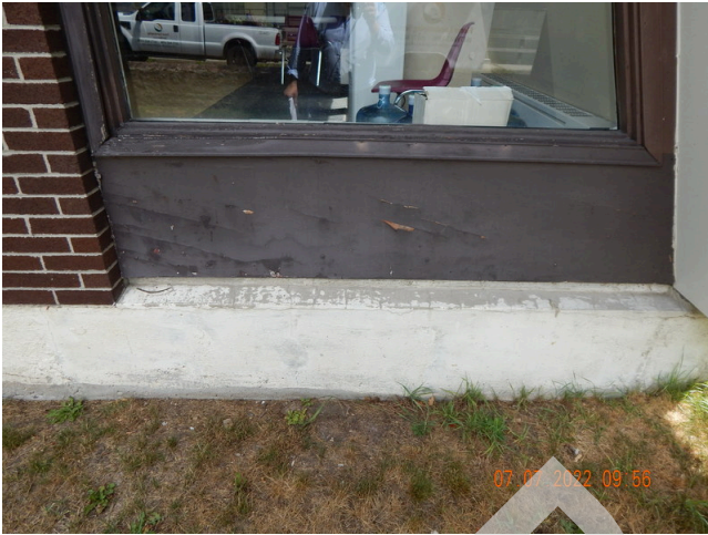
77. Sidewall System: Typical damaged or weathered wood trim found throughout the community building. (Non-Critical Repair)
