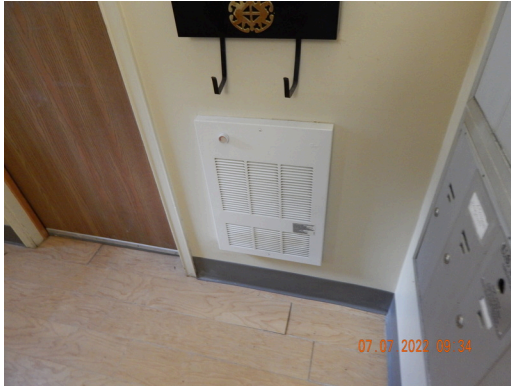
HVAC Systems: Typical electric in-wall heater found in common areas throughout the site.
