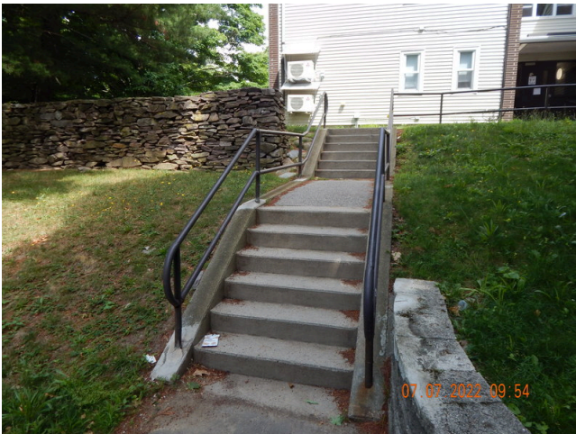
23. Flatwork (Walks, Plazas, Terraces, Patios): Concrete steps with steel handrails found at the property.
