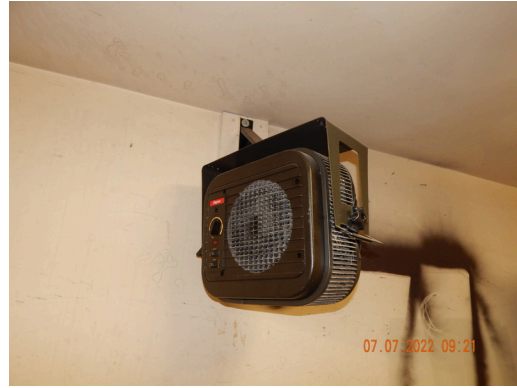
HVAC Systems: Typical electric ceiling mounted heater found in common areas throughout the site.
