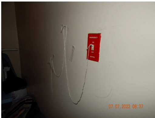
Life & Fire Safety: Typical emergency pull cord throughout the site.
