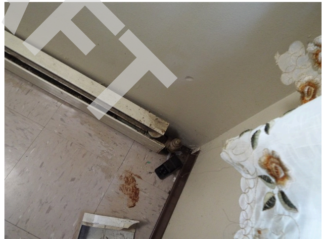
52. 1-bed-1-bath - unit 6 - baseboard heat cover condition (Non-Critical Repair)
