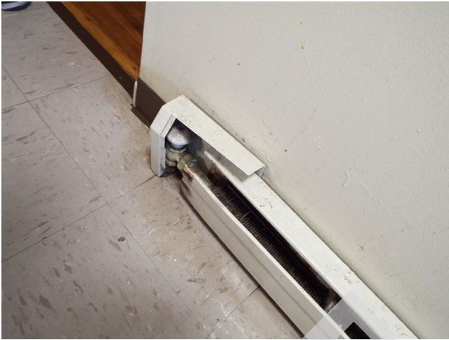
53. 1-bed-1-bath - unit 6 - baseboard heat cover condition (Non-Critical Repair)
