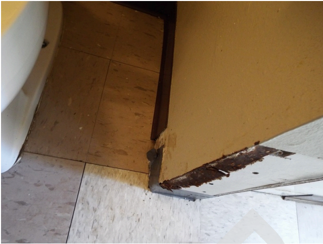
45. 1-bed-1-bath - unit 6 - wall condition (Non-Critical Repair)
