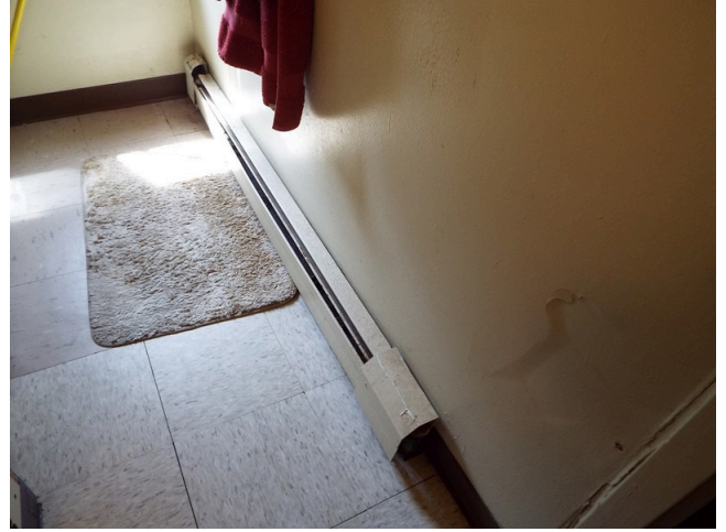
42. 1-bed-1-bath - unit 6 - baseboard heat cover condition (Non-Critical Repair)
