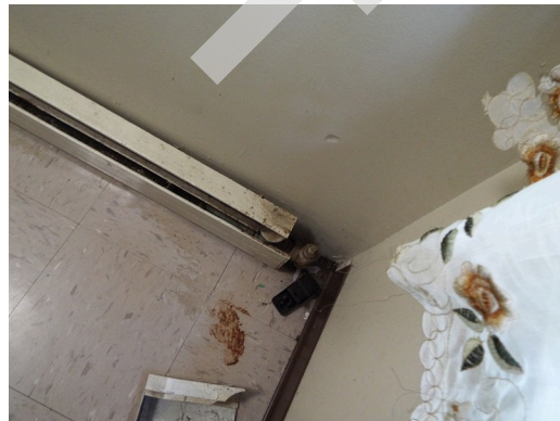
1-bed-1-bath - unit 6 - baseboard heat cover condition (Non-Critical Repair)
