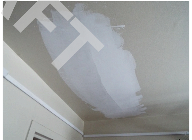
88. 1-bed-1-bath - unit 2 - ceiling condition (Non-Critical Repair)
