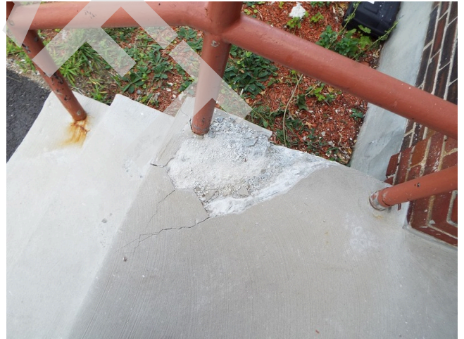
20. Building 13 entry - concrete step spalling (Critical Repair)
