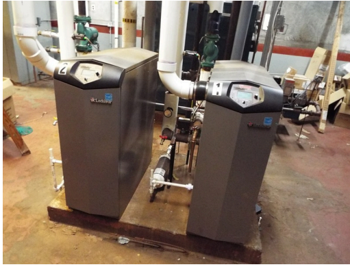
Heating hot water boilers (newer)
