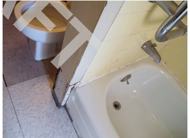
44. 1-bed-1-bath - unit 6 - wall condition (Non-Critical Repair)
