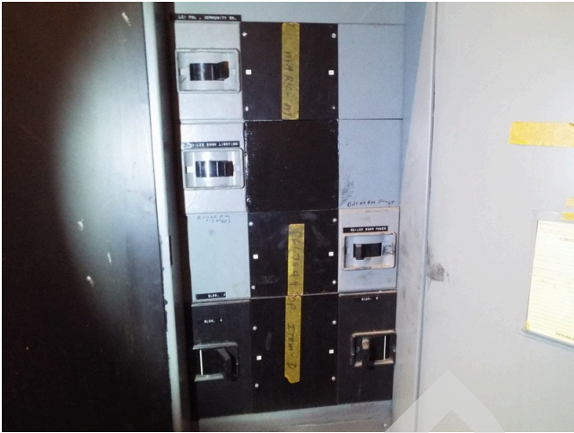
61. Main electrical panel - boiler room
