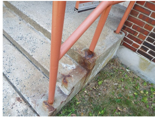
Handrail post base condition - building 15 (Critical Repair)
