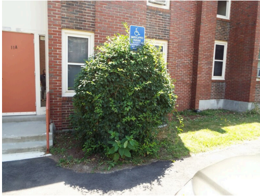
Accessible parking lacks van sign (Critical Repair)
