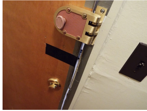
1-bed-1-bath - unit 6 - door gap (Non-Critical Repair)
