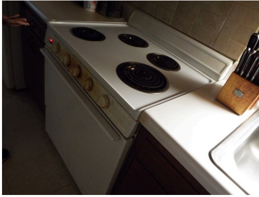
1-bed-1-bath - unit 38 - range malfunction (Critical Repair)
