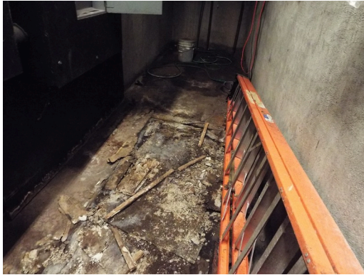
Boiler room - moisture condition (Non-Critical Repair)
