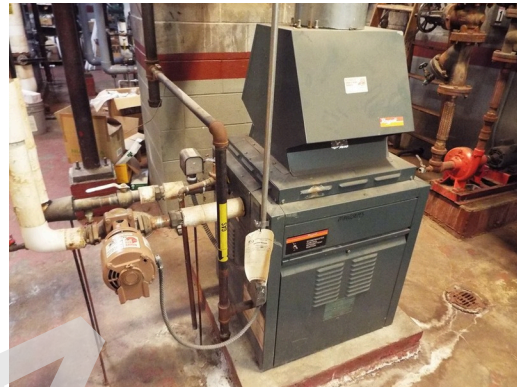
Domestic hot water boiler
