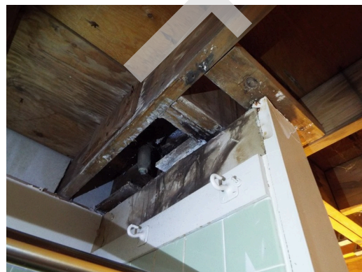
1-bed-1-bath - unit 15 - ceiling condition (Non-Critical Repair)
