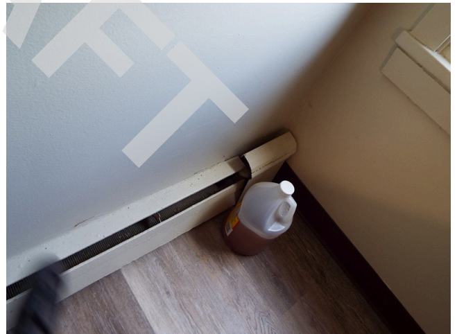
136. 1-bed-1-bath - unit 22 - baseboard heat cover condition (Non-Critical Repair)
