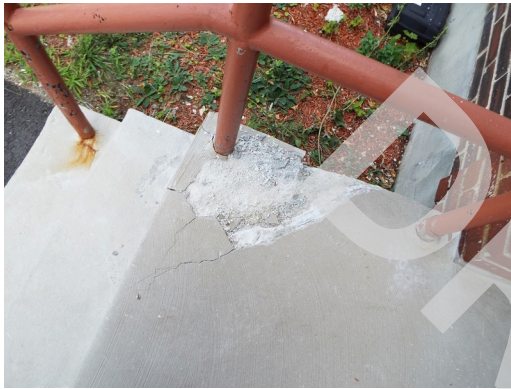
Building 13 entry - concrete step spalling (Critical Repair)
