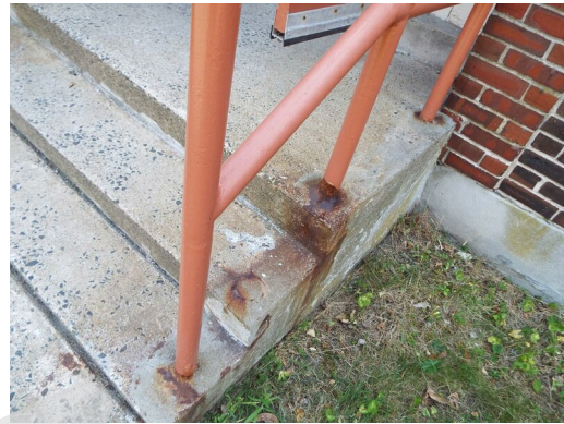
Handrail post base condition - building 15 (Critical Repair)
