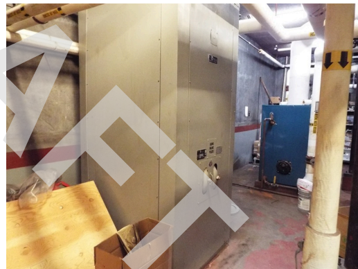
Domestic hot water vertical cabinet storage tank
