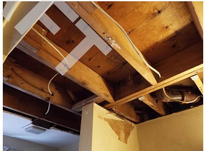
116. 1-bed-1-bath - unit 15 - ceiling condition (Non-Critical Repair)
