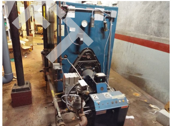
56. Heating hot water boiler (older)
