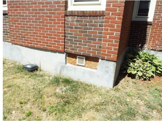
Crawlspace vent undersized (Non-Critical Repair)
