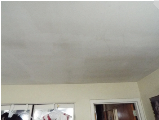
Typical unit bedroom lacks smoke detector - unit 38 (Critical Repair)
