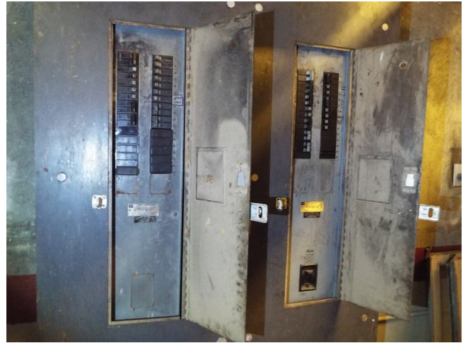
62. Electrical subpanels - boiler room
