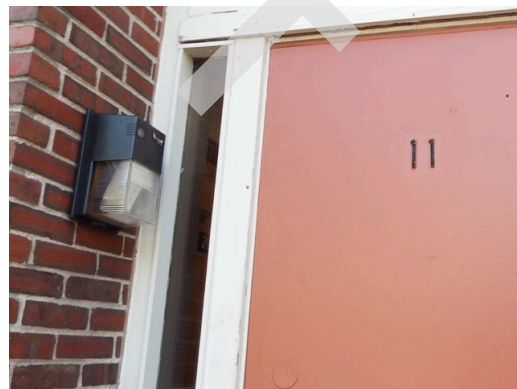
Building mounted lighting
