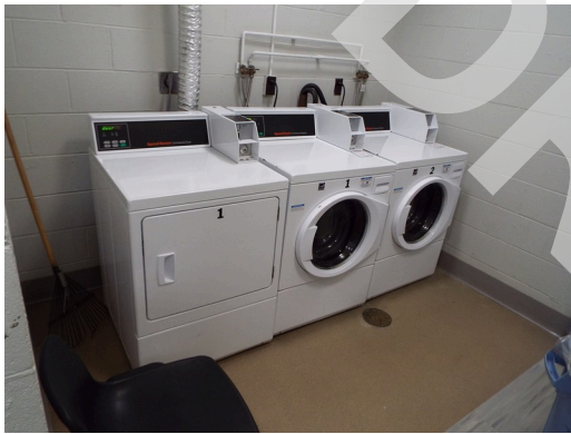
Community room - washer lacks front controls (Critical Repair)
