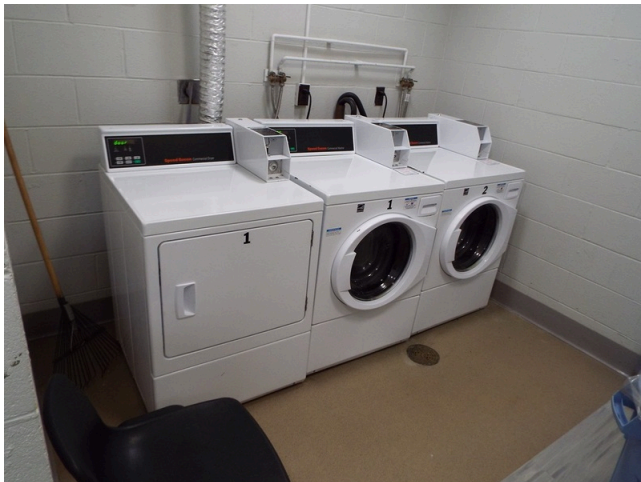
79. Community room - washer lacks front controls (Critical Repair)
