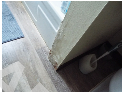
1-bed-1-bath - unit 5 - bed-1-bath - wall condition (Non-Critical Repair)
