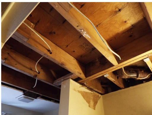
1-bed-1-bath - unit 15 - ceiling condition (Non-Critical Repair)
