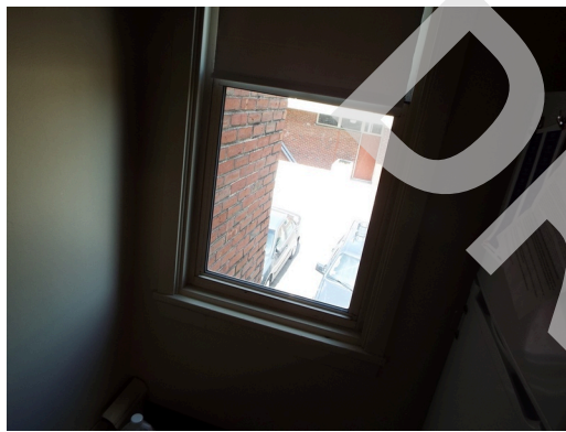
1-bed-1-bath - unit 22 - missing screen (Non-Critical Repair)
