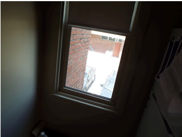
135. 1-bed-1-bath - unit 22 - missing screen (Non-Critical Repair)
