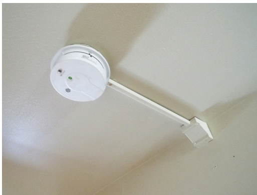
Typical hall smoke detector
