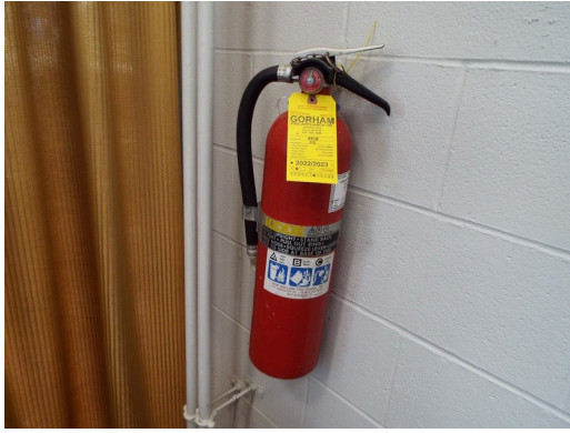
Fire extinguisher - community room
