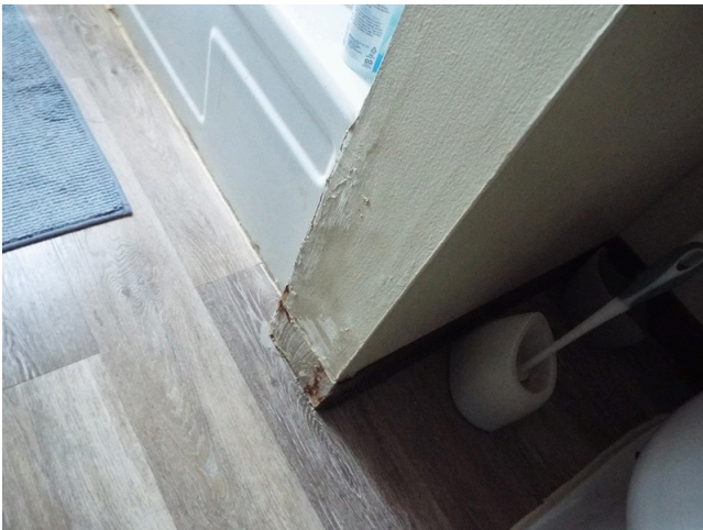
103. 1-bed-1-bath - unit 5 -bed-1-bath - wall condition (Non-Critical Repair)
