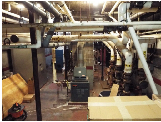
Piping - boiler room
