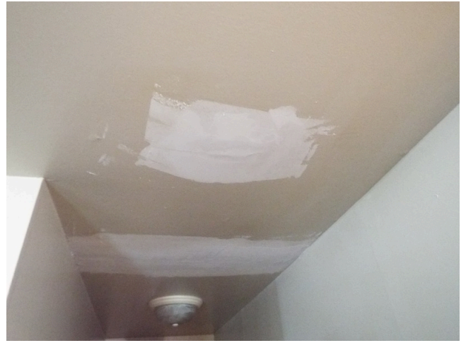
74. 1-bed-1-bath - unit 2 - ceiling condition (Non-Critical Repair)
