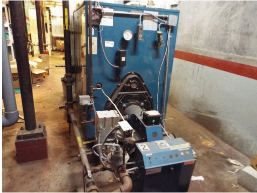
Heating hot water boiler (older)
