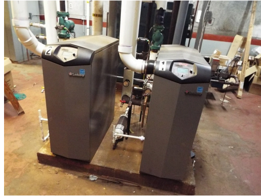
Heating hot water boilers (newer)
