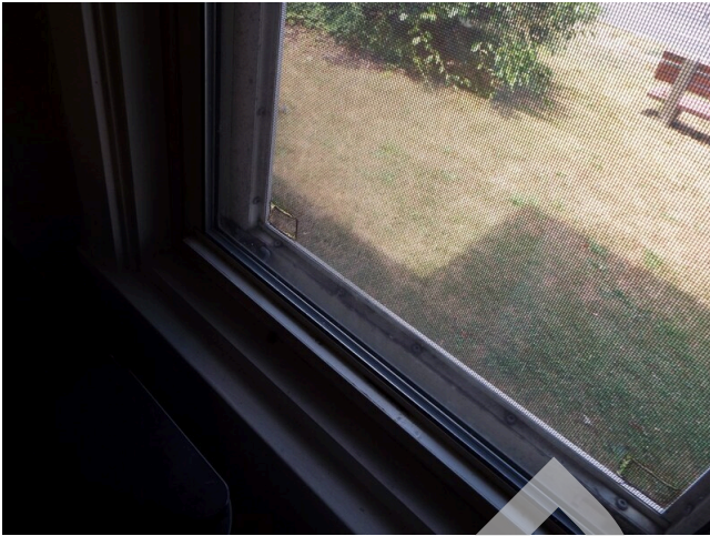
121. 1-bed-1-bath - unit 27 - screen damage (Non-Critical Repair)
