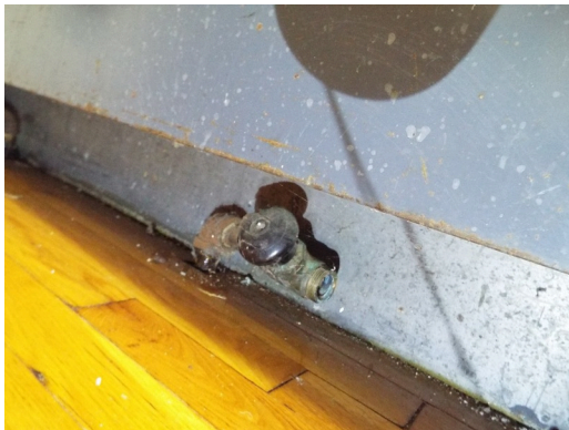
Vestibule heater disconnected - building 7 (Non-Critical Repair)
