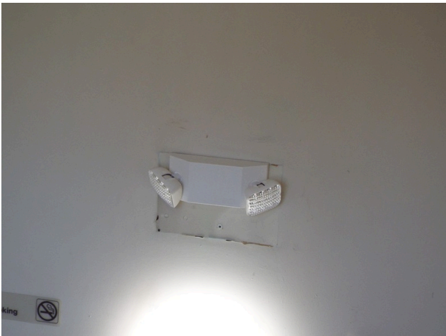
67. Interior stair - building 15
