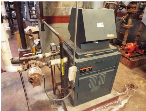
Domestic hot water boiler
