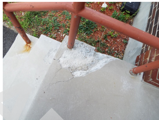
Building 13 entry - concrete step spalling (Critical Repair)
