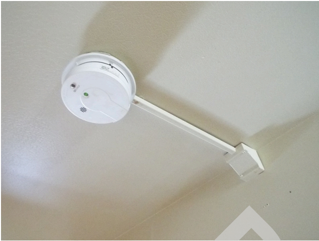
69. Typical hall smoke detector
