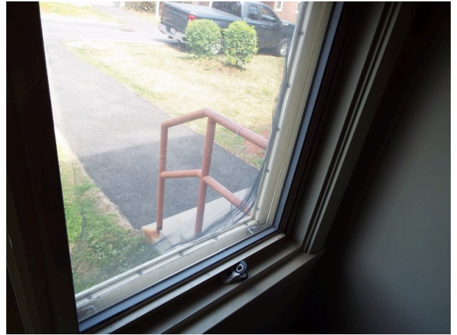
122. 1-bed-1-bath - unit 27 - screen damage (Non-Critical Repair)
