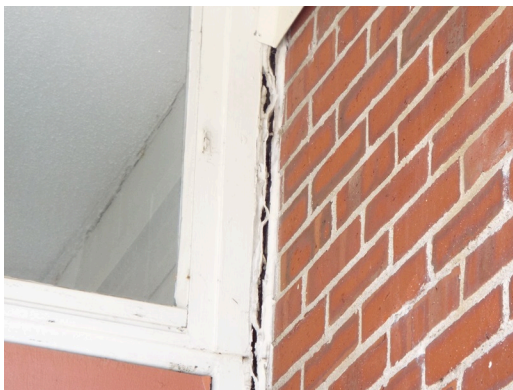
Sealant condition - community center rear door (Non-Critical Repair)
