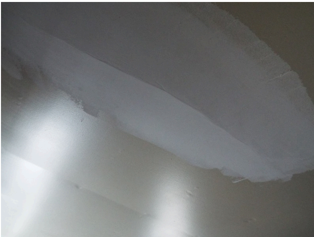
87. 1-bed-1-bath - unit 2 - ceiling condition (Non-Critical Repair)
