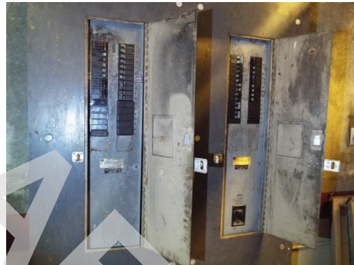
Electrical subpanels - boiler room
