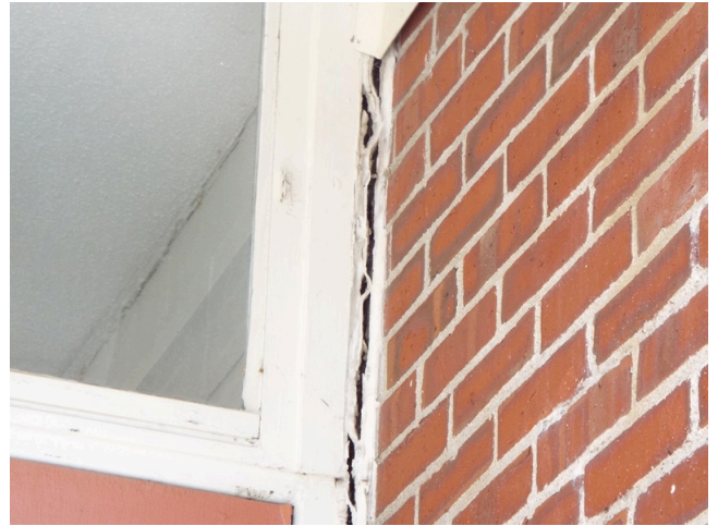
42. Sealant condition - community center rear door (Non-Critical Repair)
