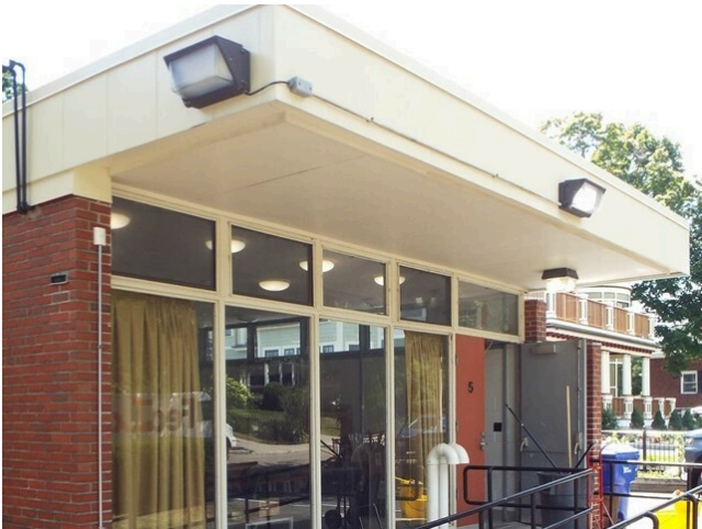
27. Building mounted lighting
