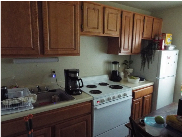
99. 1-bed-1-bath - unit 5 - range malfunction (Critical Repair)
