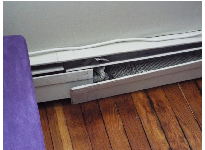
90. 1-bed-1-bath - unit 2 - baseboard heat cover condition (Non-Critical Repair)
