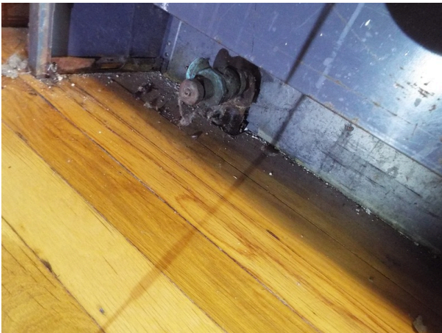
59. Vestibule heater disconnected - building 15A (Non-Critical Repair)
