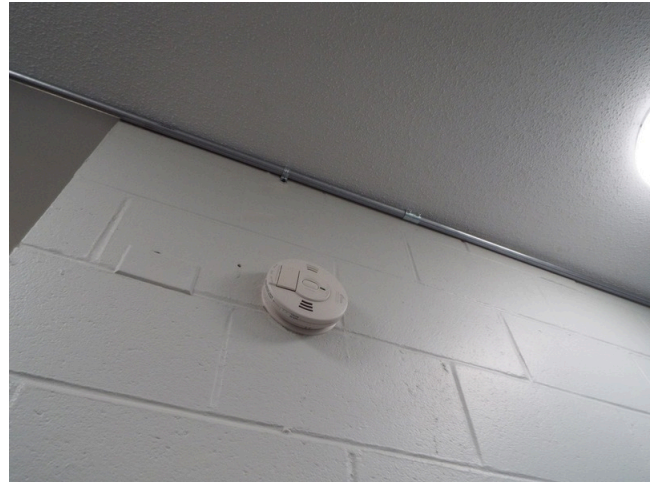
70. Community room - smoke detector
