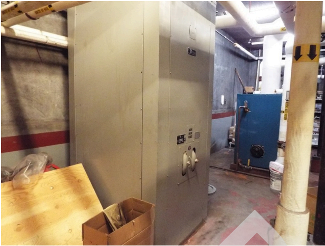
53. Domestic hot water vertical cabinet storage tank
