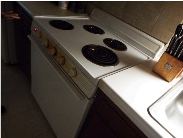
3. 1-bed-1-bath - unit 38 - range malfunction (Critical Repair)
