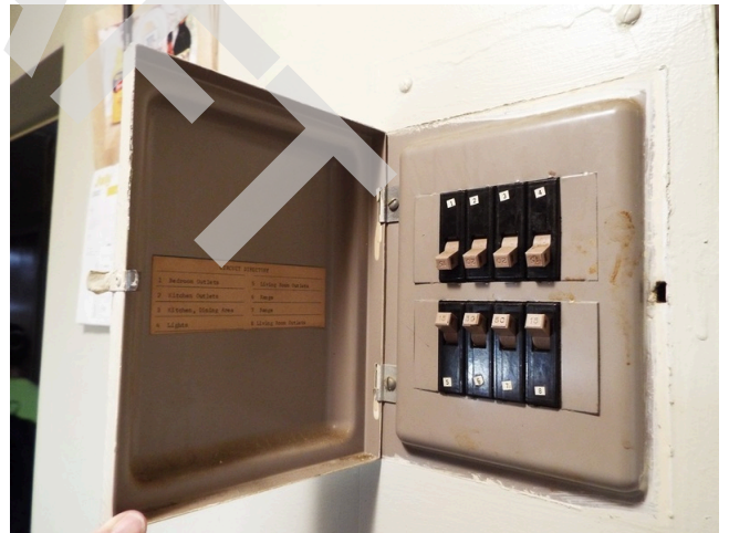
64. Typical unit electrical panel - unit 38
