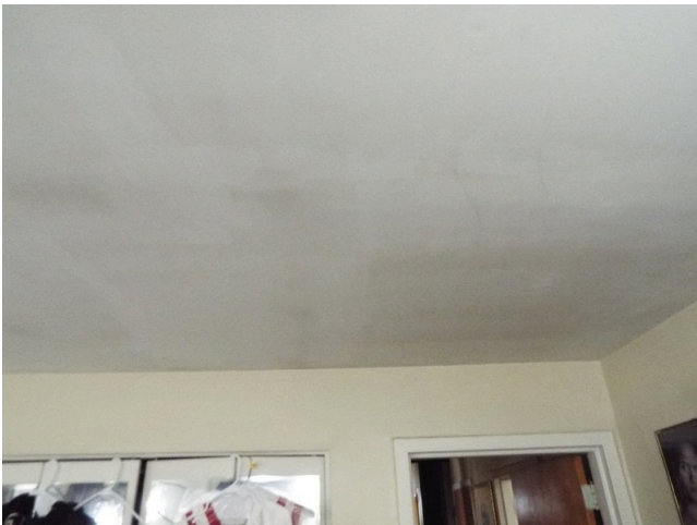
15. Typical unit bedroom lacks smoke detector - unit 38 (Critical Repair)
