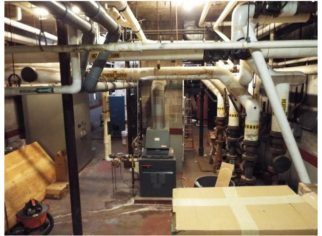
54. Piping - boiler room
