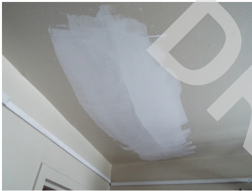
1-bed-1-bath - unit 2 - ceiling condition (Non-Critical Repair)
