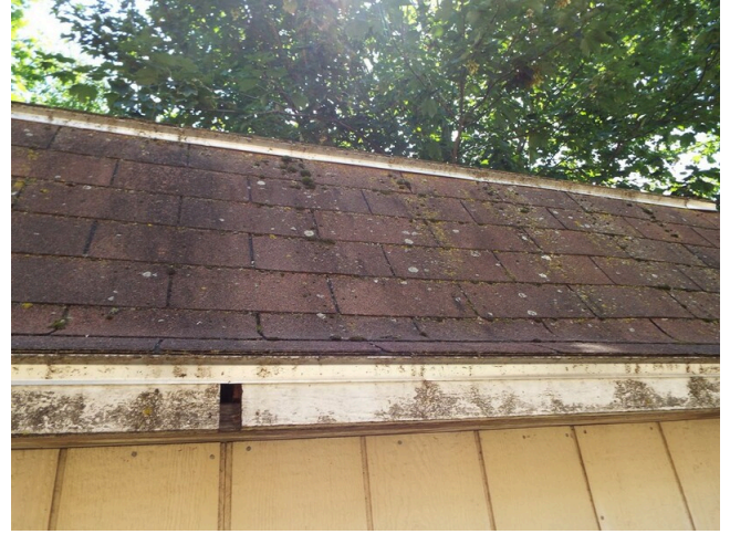
30. Utility shed fascia and roof condition (Non-Critical Repair)
