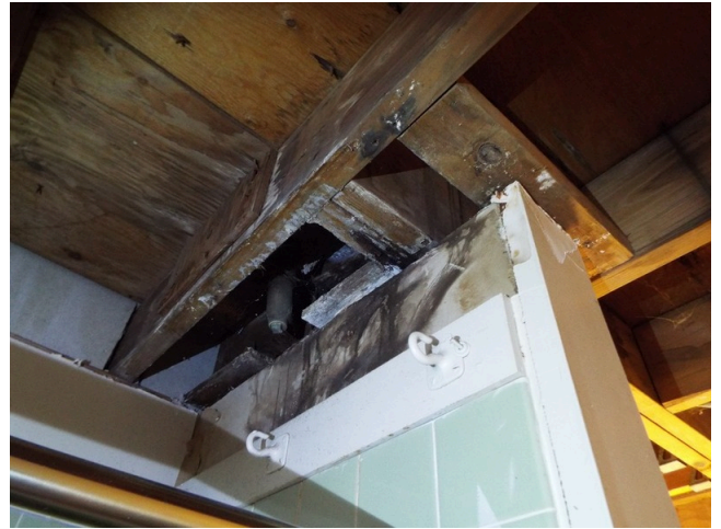
118. 1-bed-1-bath - unit 15 - ceiling condition (Non-Critical Repair)
