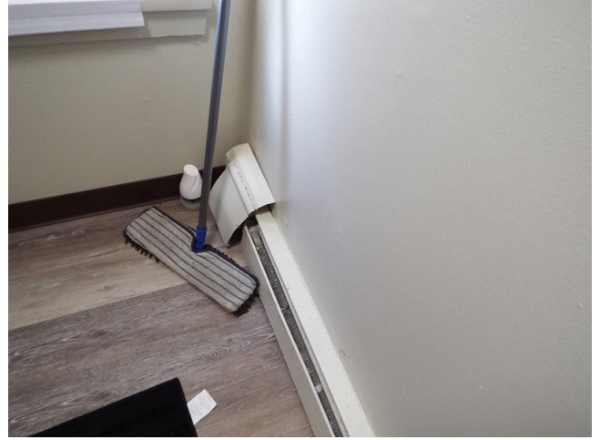
146. 1-bed-1-bath - unit 22 - baseboard heat cover condition (Non-Critical Repair)
