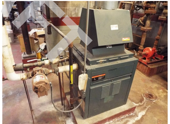
52. Domestic hot water boiler
