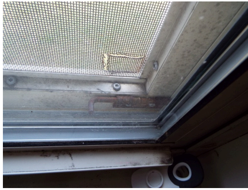
1-bed-1-bath - unit 27 - screen damage (Non-Critical Repair)
