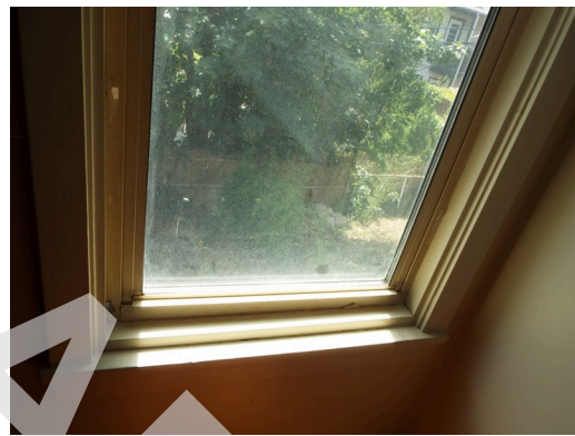
1-bed-1-bath - unit 22 - missing screen (Non-Critical Repair)
