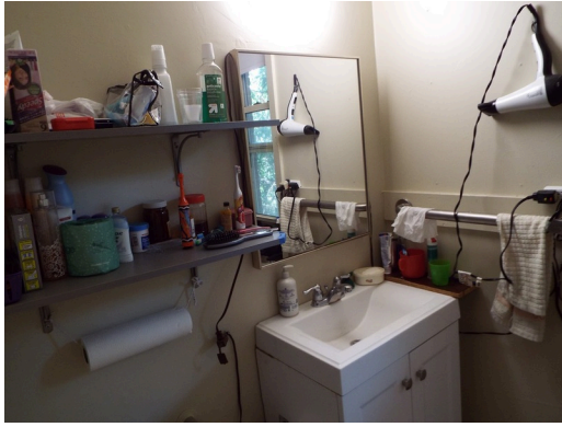
2-bed-1-bath - unit 40 - non-GFCI protected electric devices (Critical Repair)
