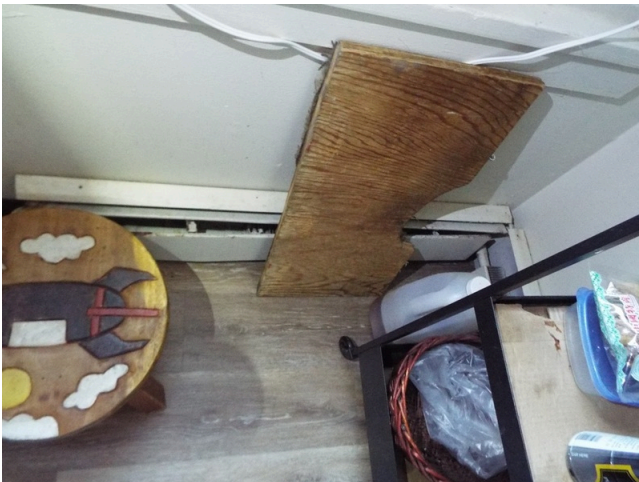
63. 2-bed-1-bath - unit 40 - baseboard heat cover condition (Non-Critical Repair)
