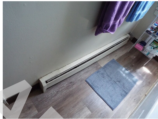
1-bed-1-bath - unit 5 - baseboard heat cover condition (Non-Critical Repair)
