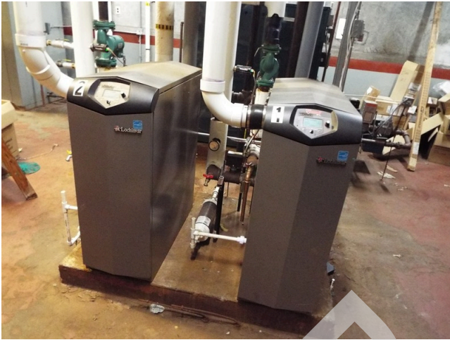
57. Heating hot water boilers (newer)
