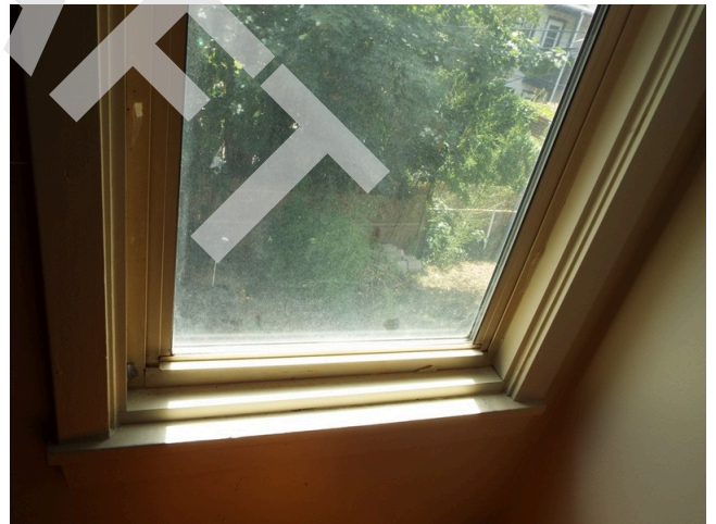
140. 1-bed-1-bath - unit 22 - missing screen (Non-Critical Repair)
