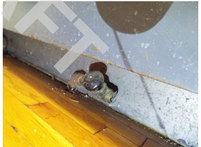
60. Vestibule heater disconnected - building 7 (Non-Critical Repair)
