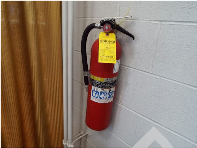
65. Fire extinguisher - community room
