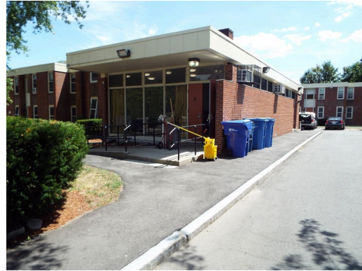
Community room entry lacks directional signage to accessible parking (Critical Repair)
