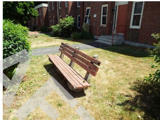
Bench condition (Non-Critical Repair)
