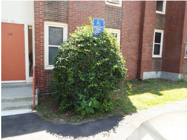
77. Accessible parking lacks van sign (Critical Repair)
