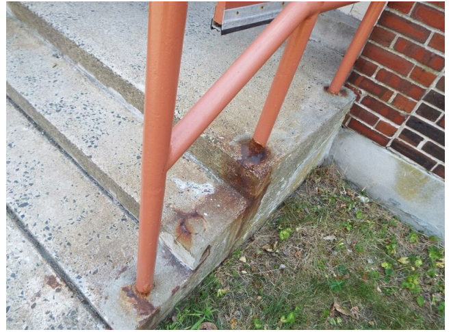
18. Handrail post base condition - building 15 (Critical Repair)
