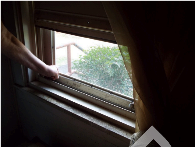
25. 1-bed-1-bath - unit 36 - inoperable screen locking device (Non-Critical Repair)
