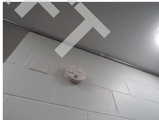
Community room - smoke detector
