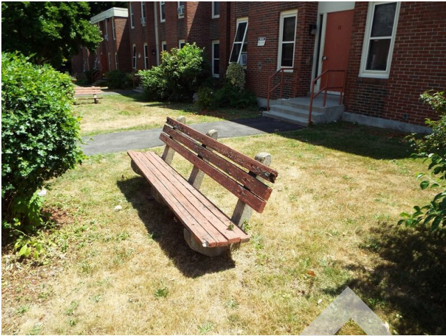
25. Bench condition (Non-Critical Repair)
