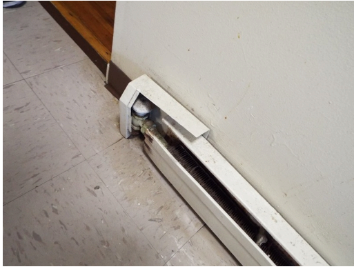
1-bed-1-bath - unit 6 - baseboard heat cover condition (Non-Critical Repair)
