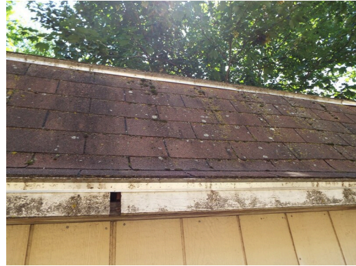
Utility shed fascia and roof condition (Non-Critical Repair)
