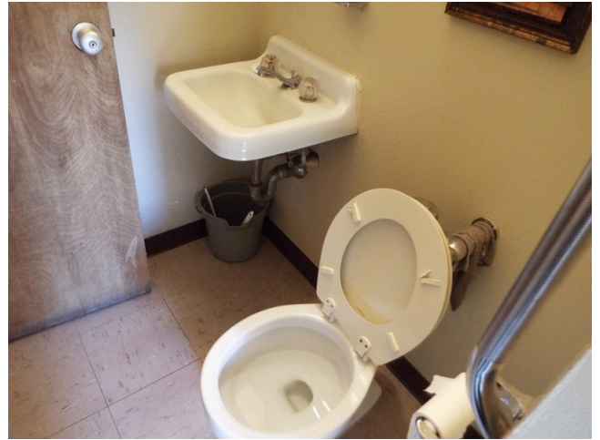
46. 1-bed-1-bath - unit 6 - bathroom fixtures
