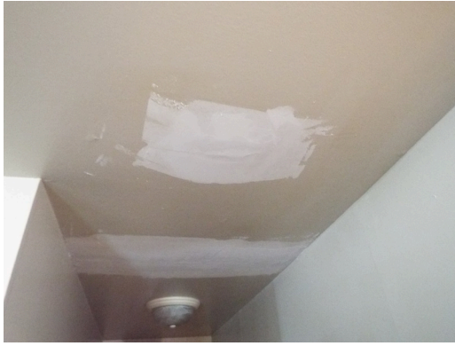
1-bed-1-bath - unit 2 - ceiling condition (Non-Critical Repair)
