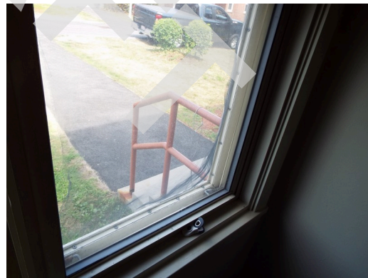
1-bed-1-bath - unit 27 - screen damage (Non-Critical Repair)
