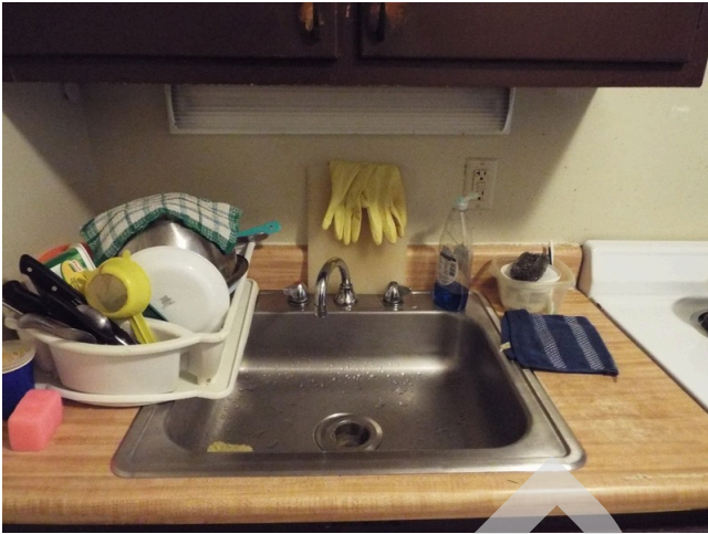
113. 1-bed-1-bath - unit 15 - typical kitchen GFCI receptacle
