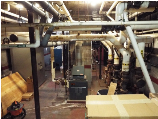
Piping - boiler room
