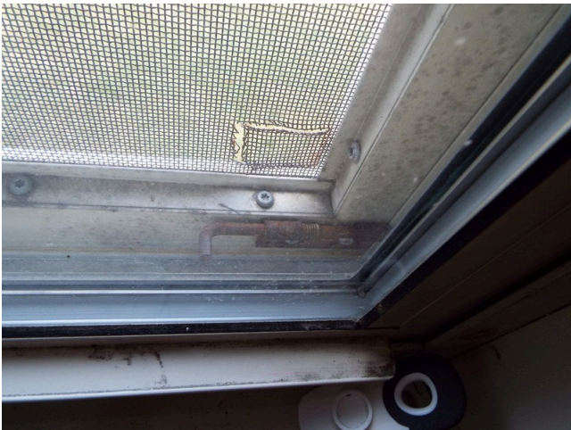
123. 1-bed-1-bath - unit 27 - screen damage (Non-Critical Repair)
