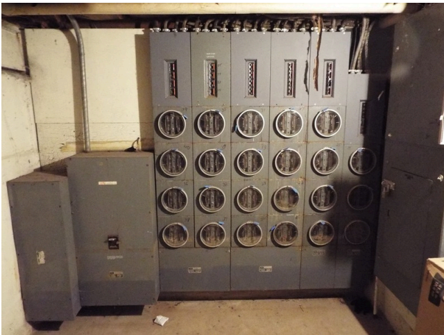
63. Meter sockets - electric room, stab lock breakers (Critical Repair)
