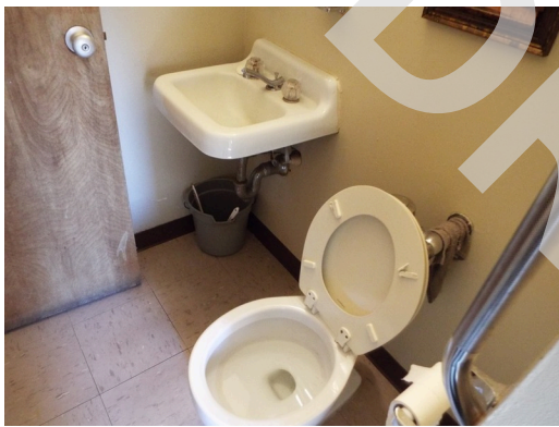
1-bed-1-bath - unit 6 - bathroom fixtures
