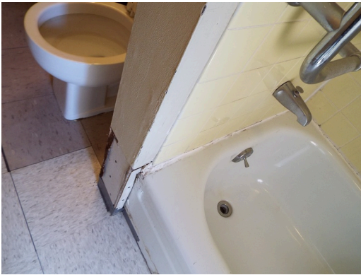
1-bed-1-bath - unit 6 - wall condition (Non-Critical Repair)
