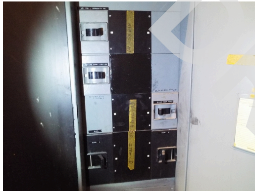
Main electrical panel - boiler room
