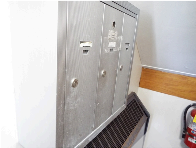
81. Mailbox condition - building 5A
