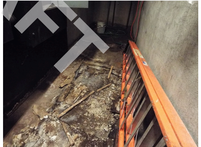
32. Boiler room - moisture condition (Non-Critical Repair)
