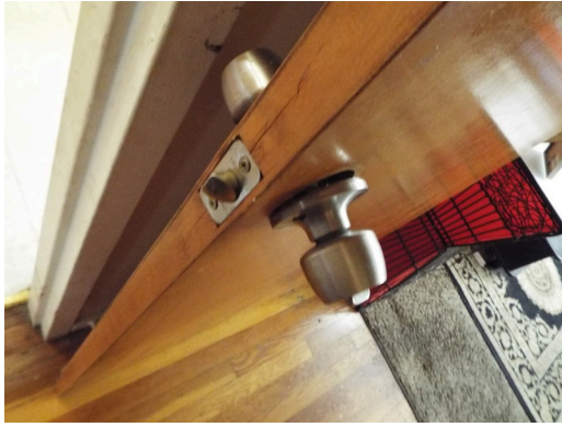
1-bed-1-bath - unit 38 - door lock condition (Critical Repair)
