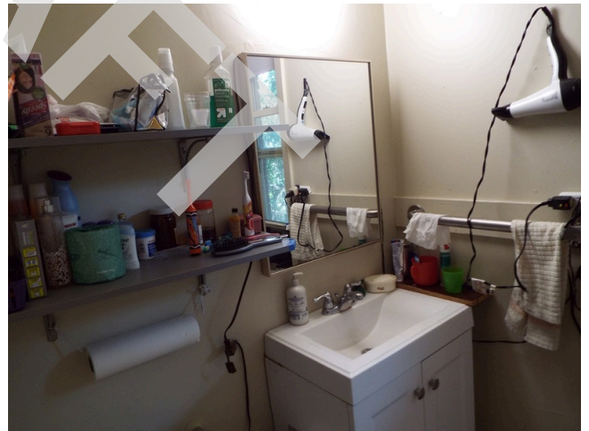
68. 2-bed-1-bath - unit 40 - non-GFCI protected electric devices (Critical Repair)
