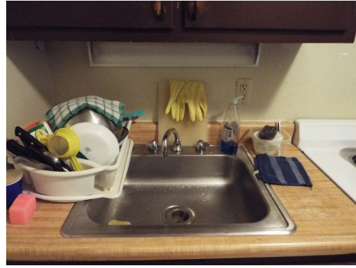
1-bed-1-bath - unit 15 - typical kitchen GFCI receptacle
