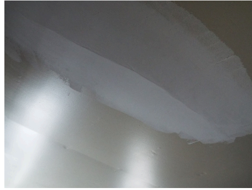
1-bed-1-bath - unit 2 - ceiling condition (Non-Critical Repair)
