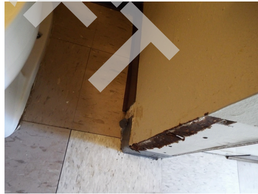
1-bed-1-bath - unit 6 - wall condition (Non-Critical Repair)
