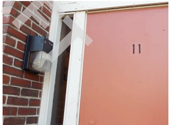
28. Building mounted lighting
