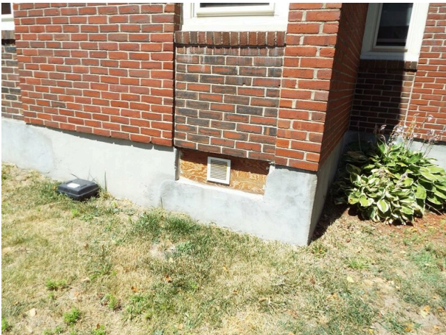
35. Crawlspace vent undersized (Non-Critical Repair)
