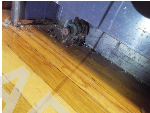
Vestibule heater disconnected - building 15A (Non-Critical Repair)
