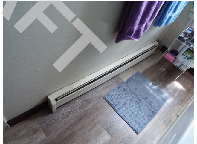
104. 1-bed-1-bath - unit 5 - baseboard heat cover condition (Non-Critical Repair)
