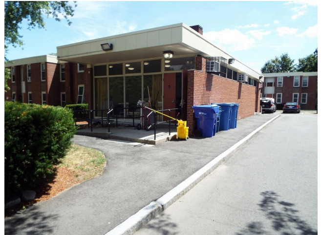
78. Community room entry lacks directional signage to accessible parking (Critical Repair)
