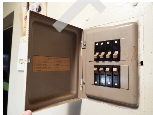
Typical unit electrical panel - unit 38
