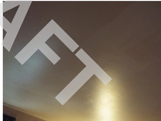
Typical unit bedroom lacks smoke detector - unit 36 (Critical Repair)
