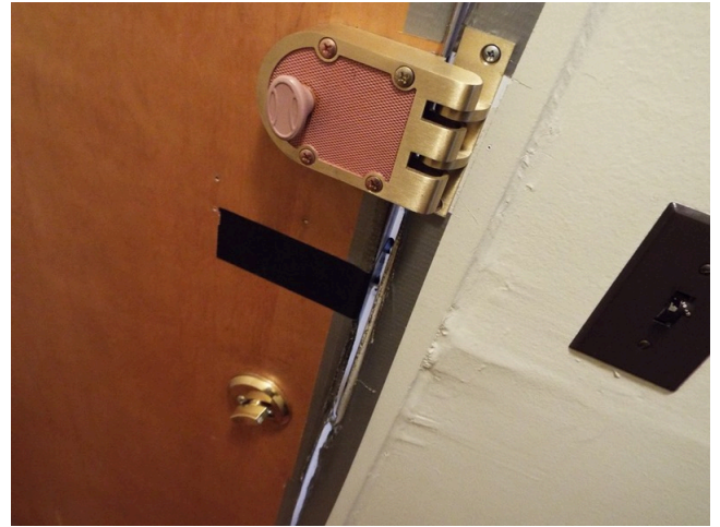
58. 1-bed-1-bath - unit 6 - door gap (Non-Critical Repair)
