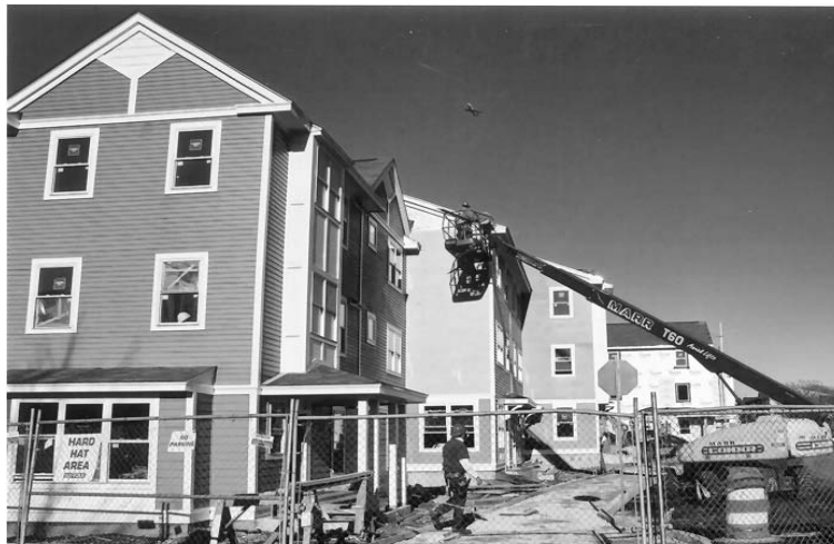
Construction is nearing completion on 133-units of affordable housing in South Boston.
