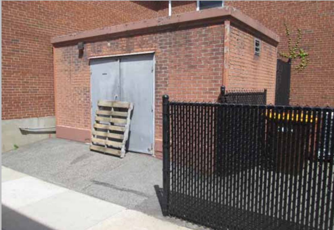
View of faded and rusted metal doors at maintenance building (Non-Critical Repairs)
