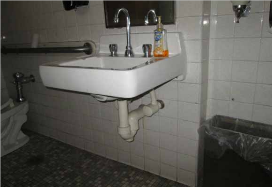
View of non-compliant sink hardware in the men’s public restroom (Critical Repair)
