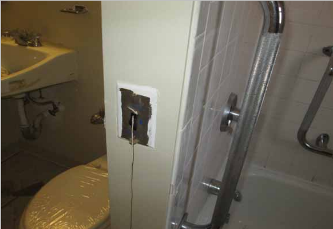
View of emergency pull cord - dwelling unit
