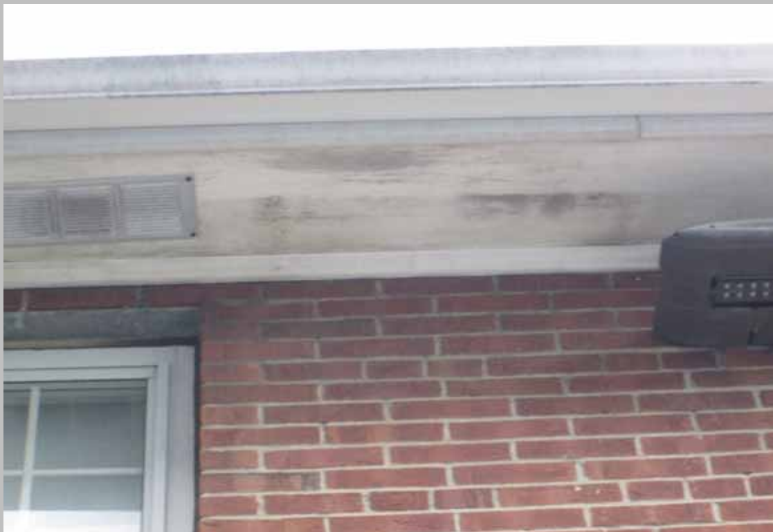
View of exterior mildew growth in need of pressure washing (Non-Critical Repair)
