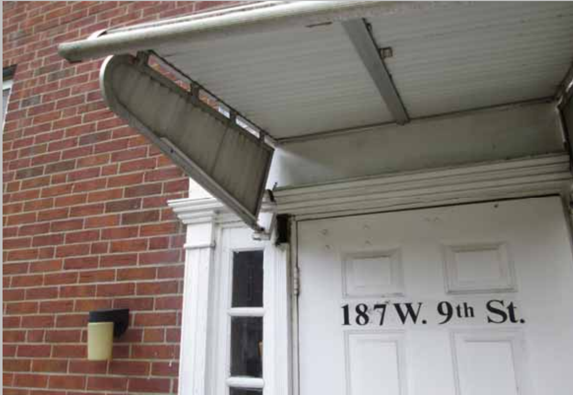
View of unsecured awning (Non-Critical Repairs)
