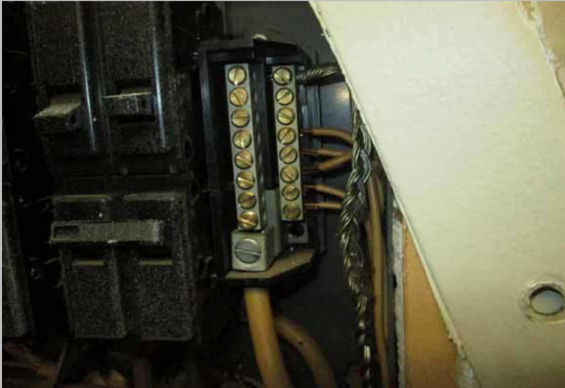
View of copper wire detail at electric breaker panel - dwelling unit
