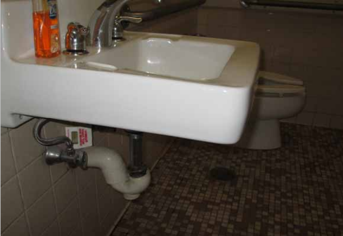
View of missing scald and abrasion protection at the women’s public restroom sink (Critical Repair)
