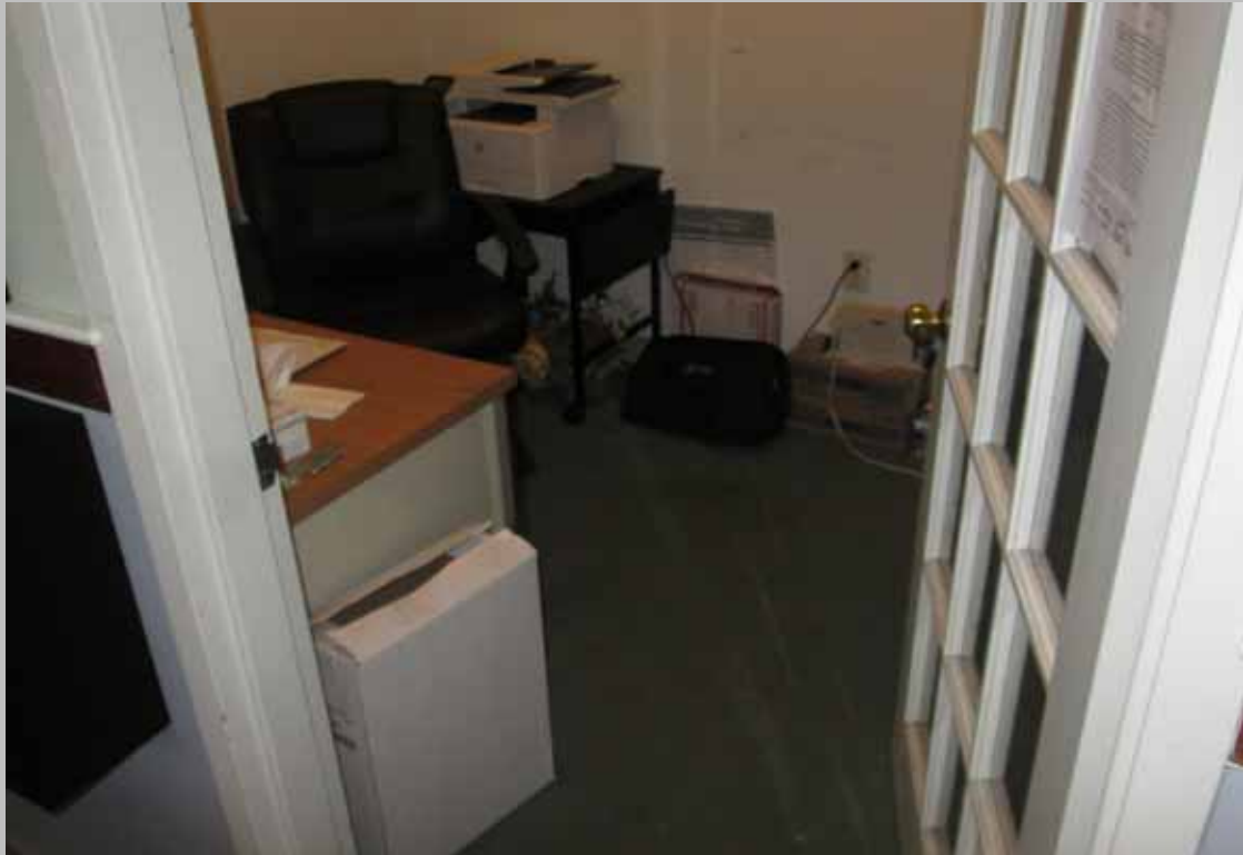
View of non-compliant knobbed hardware located at the leasing office entry door (Critical Repair)
