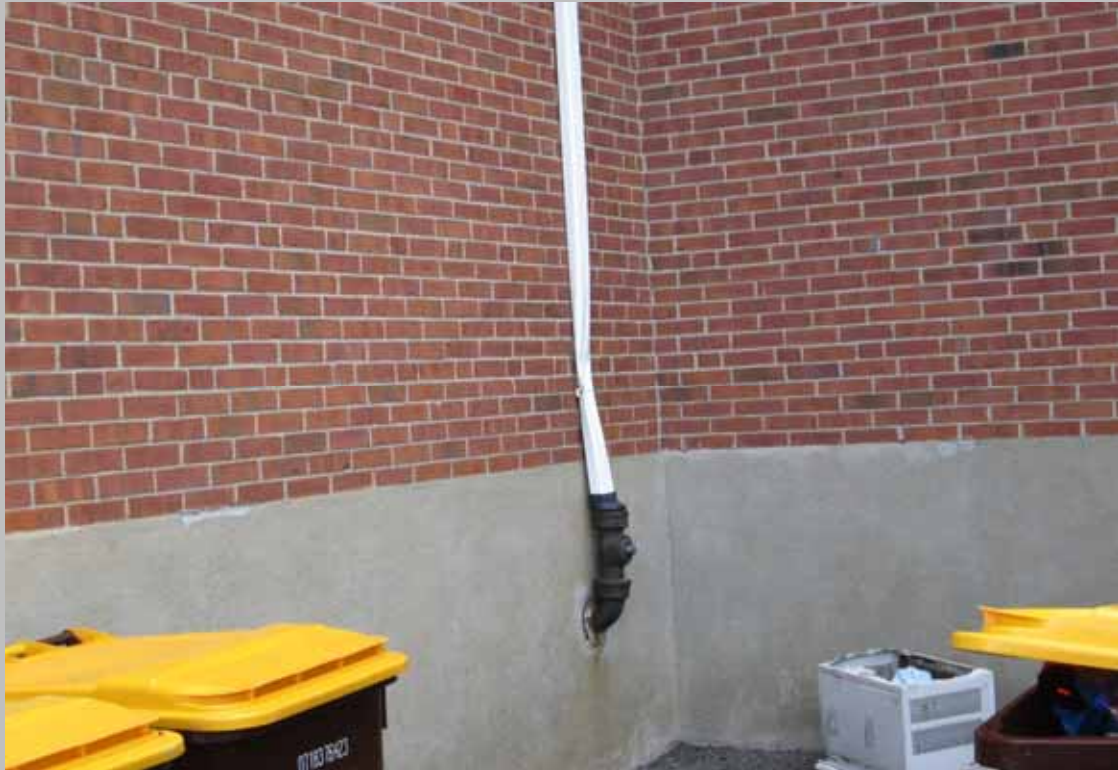
View of dented aluminum downspout (Non-Critical Repairs)
