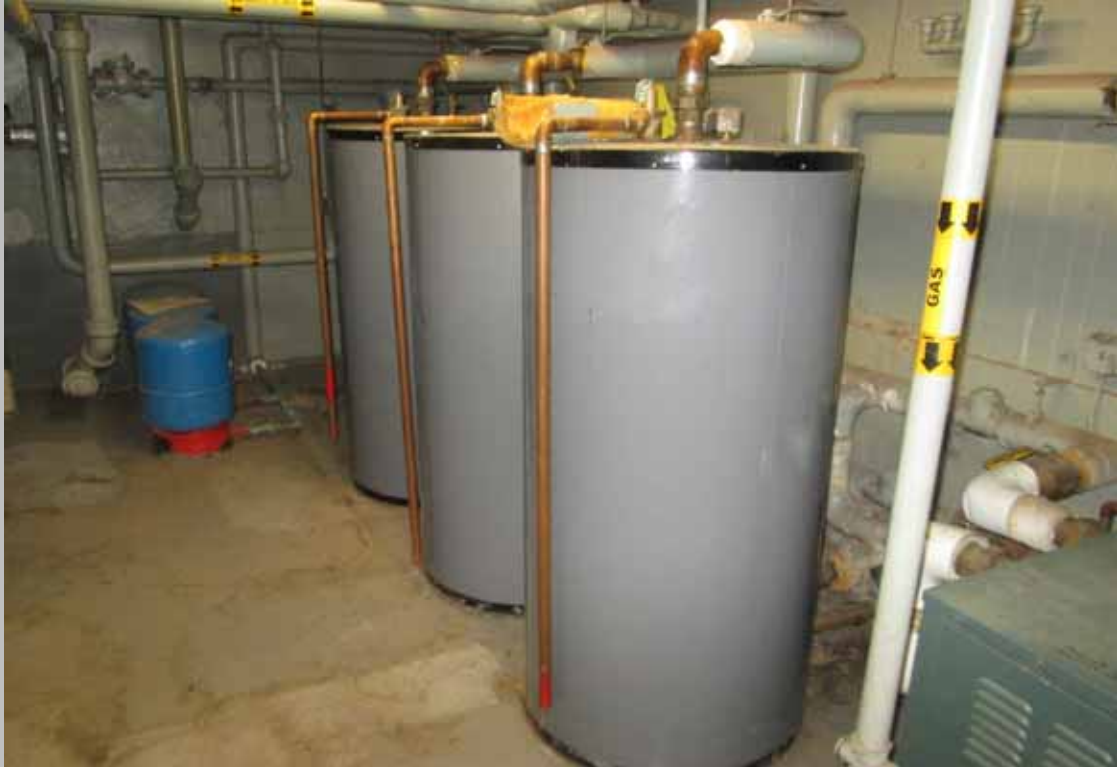
View of DHW storage tanks
