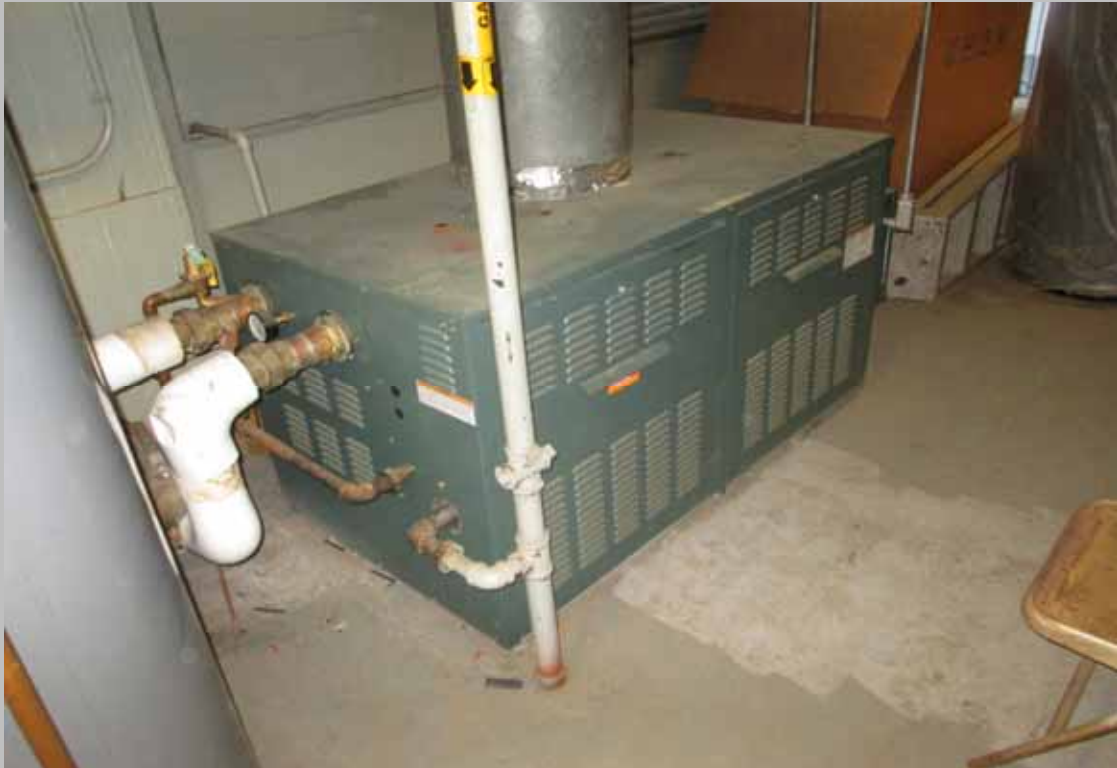
View of DHW boiler
