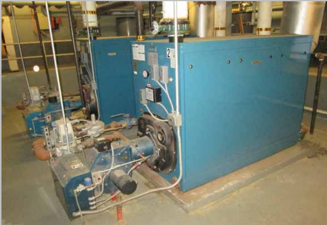
View of heating boilers
