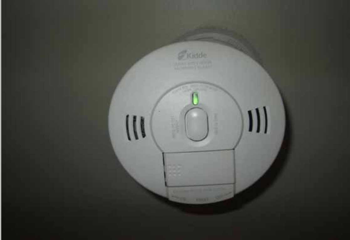
View of smoke detector - dwelling unit
