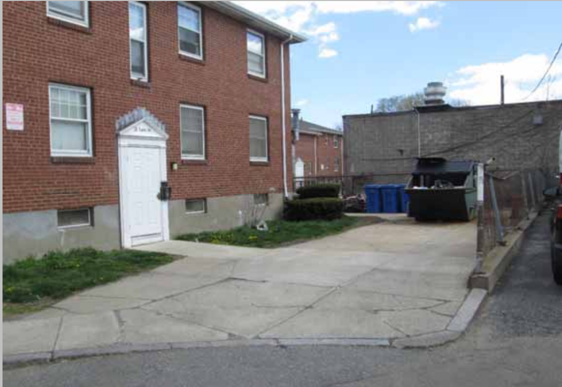
View of a potential trip hazard outside of the entry to 21 Lark Street - Critical Repair
