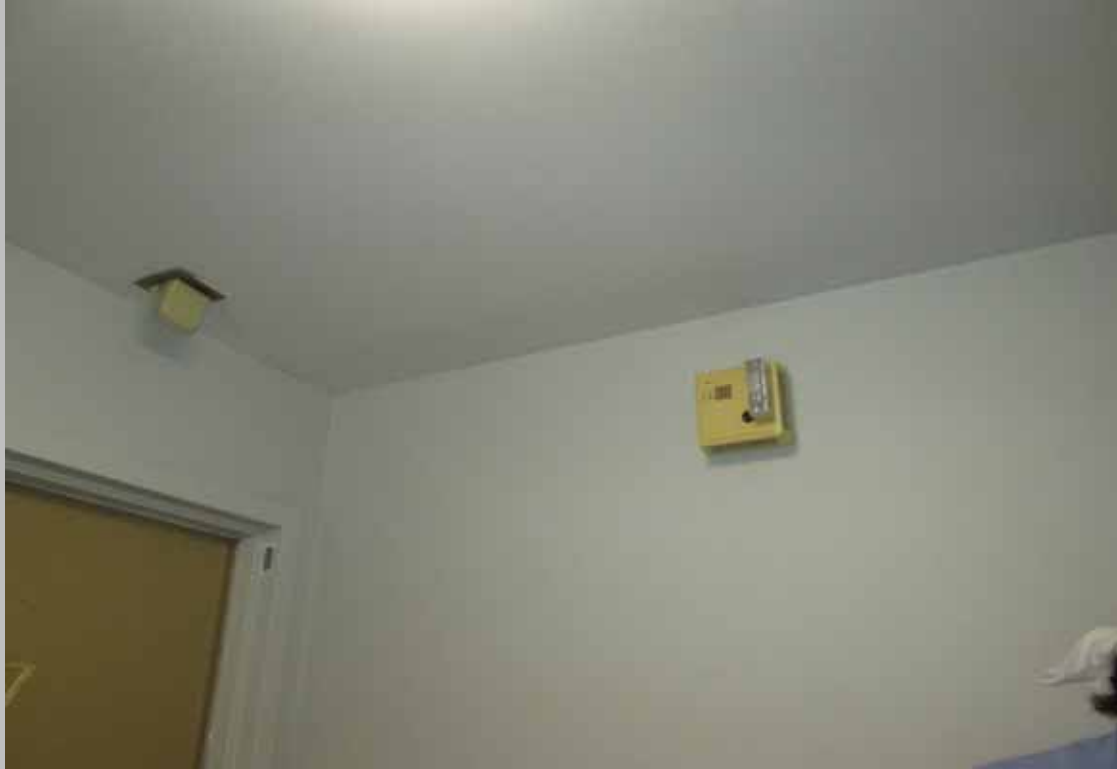
View of fire alarm in common areas
