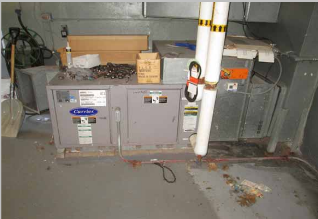
View of HVAC equipment
