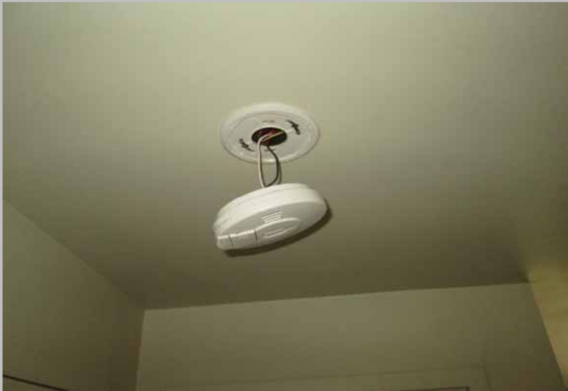
View of a typical smoke detector - dwelling unit
