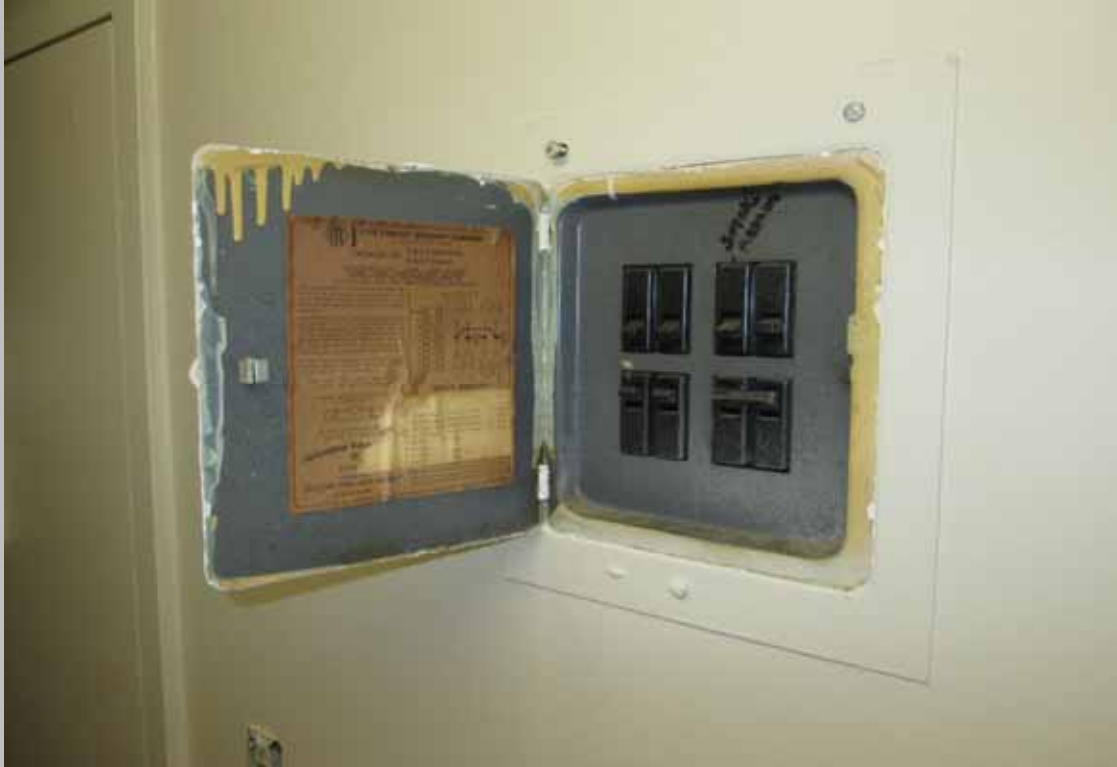
View of electric breaker panel - dwelling unit
