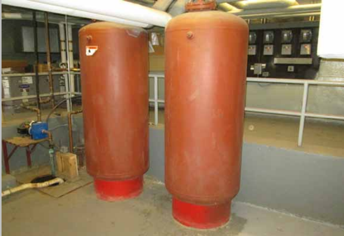
View of expansion tanks
