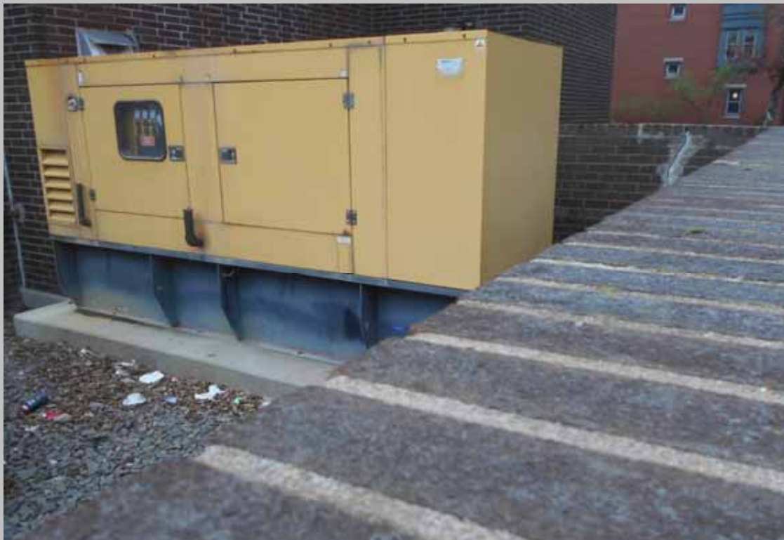
View of generator
