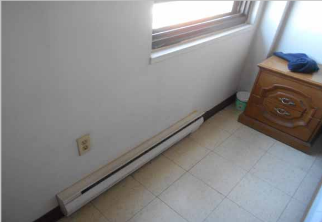
View of an electric baseboard heater – dwelling unit
