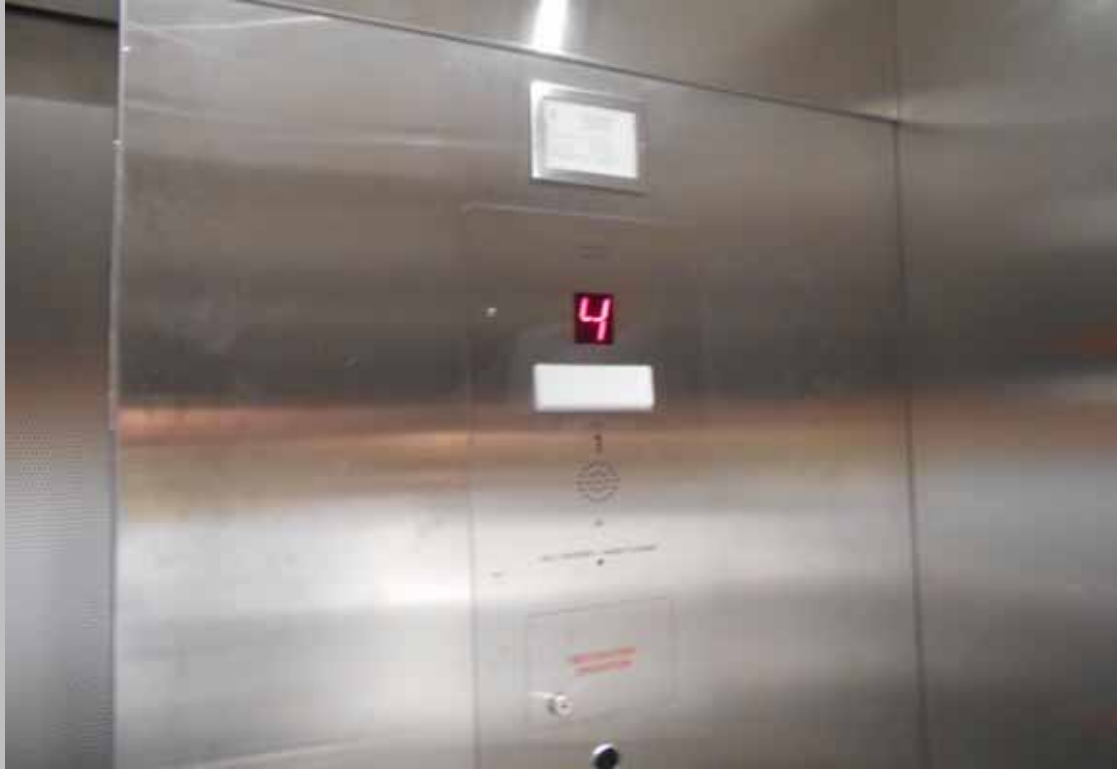
View of an elevator cab interior
