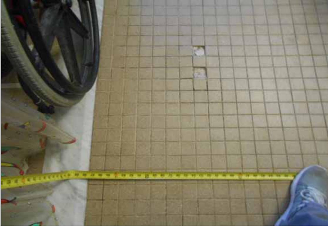
View of damaged ceramic tile bathroom flooring in unit 407 (Non-Critical Repair)
