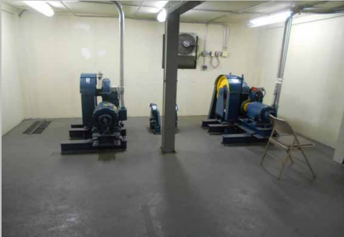
View of elevator equipment
