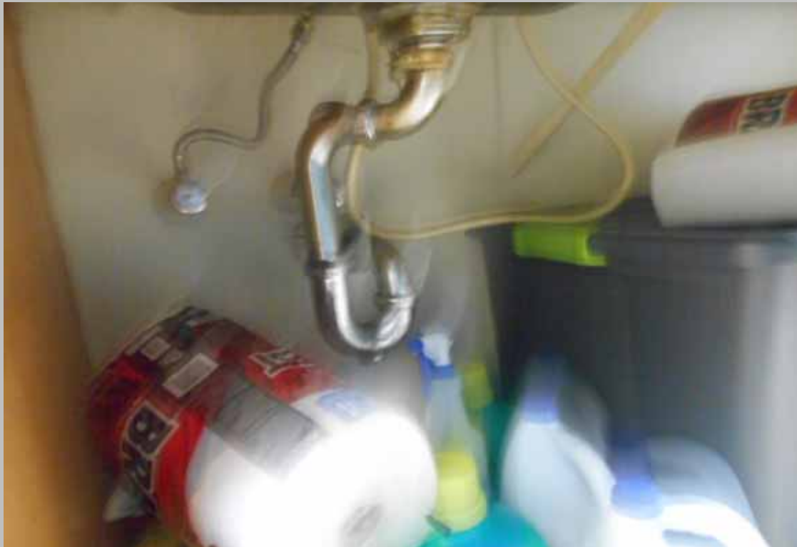
The designated handicapped dwelling unit kitchen sinks do not feature scald and abrasion protection at under-sink plumbing (Critical Repair)
