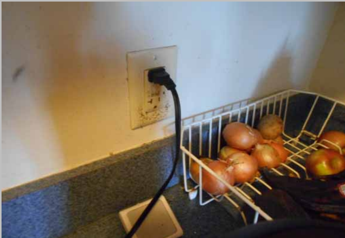
View of GFCI electrical outlet – dwelling unit
