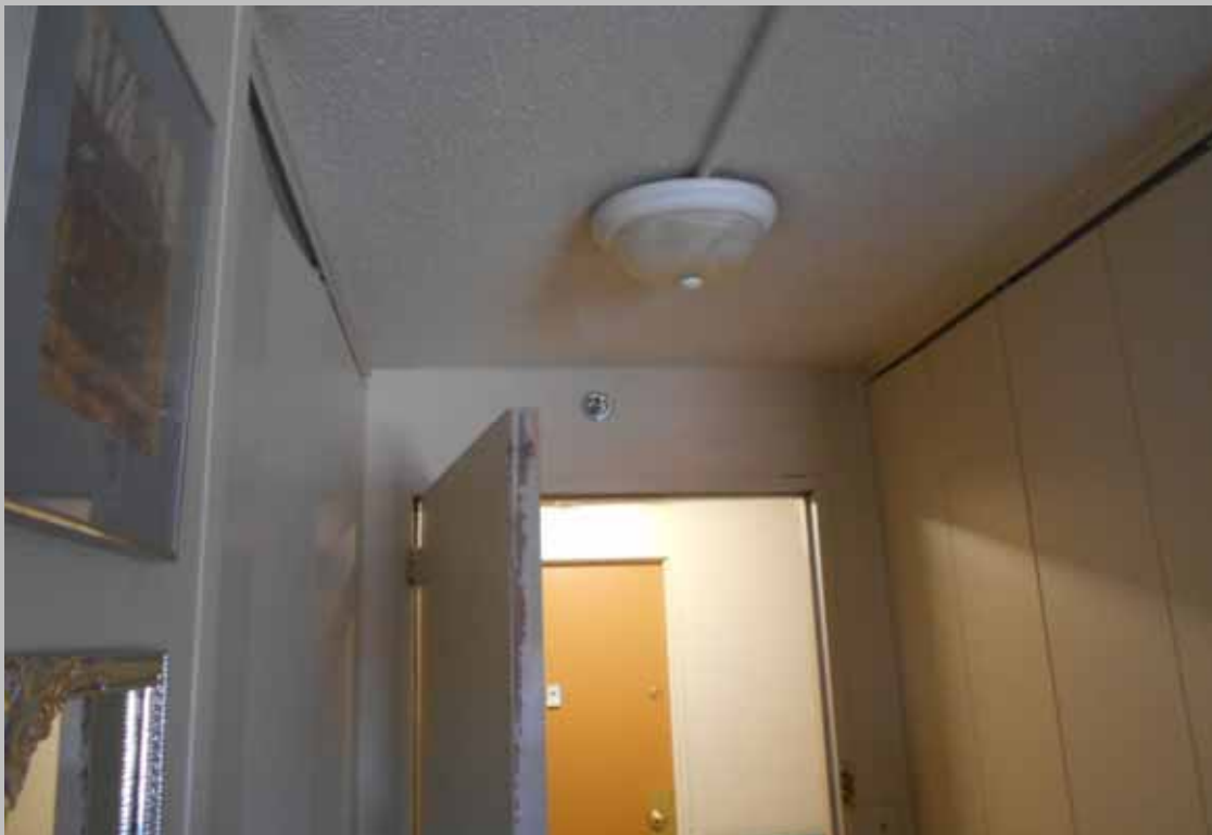
View of fire sprinkler head – dwelling unit
