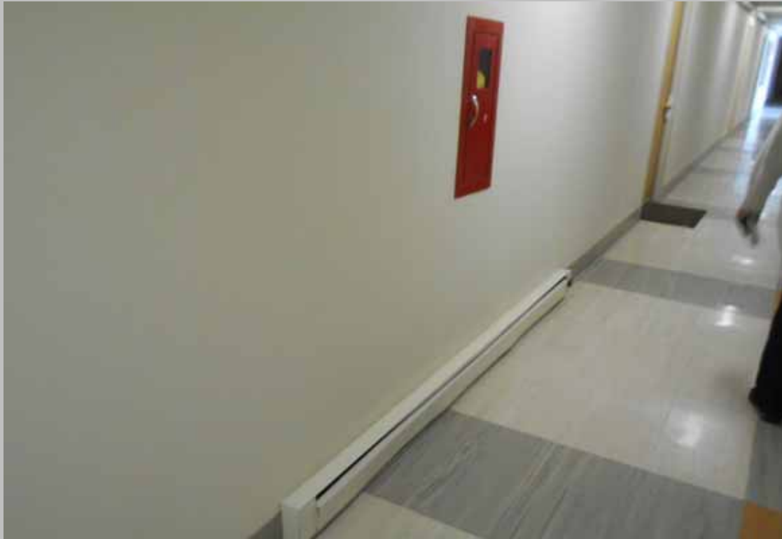
View of a common area electric baseboard heater
