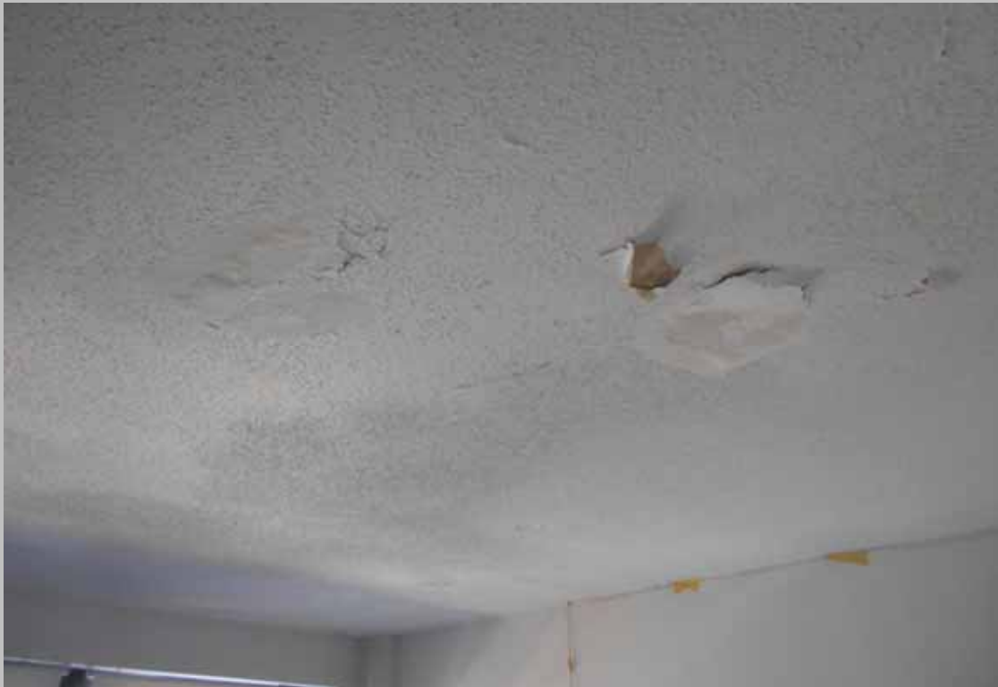
View of an example of a dwelling unit GWB in need of repair and re-painting (Non-Critical RepairS)
