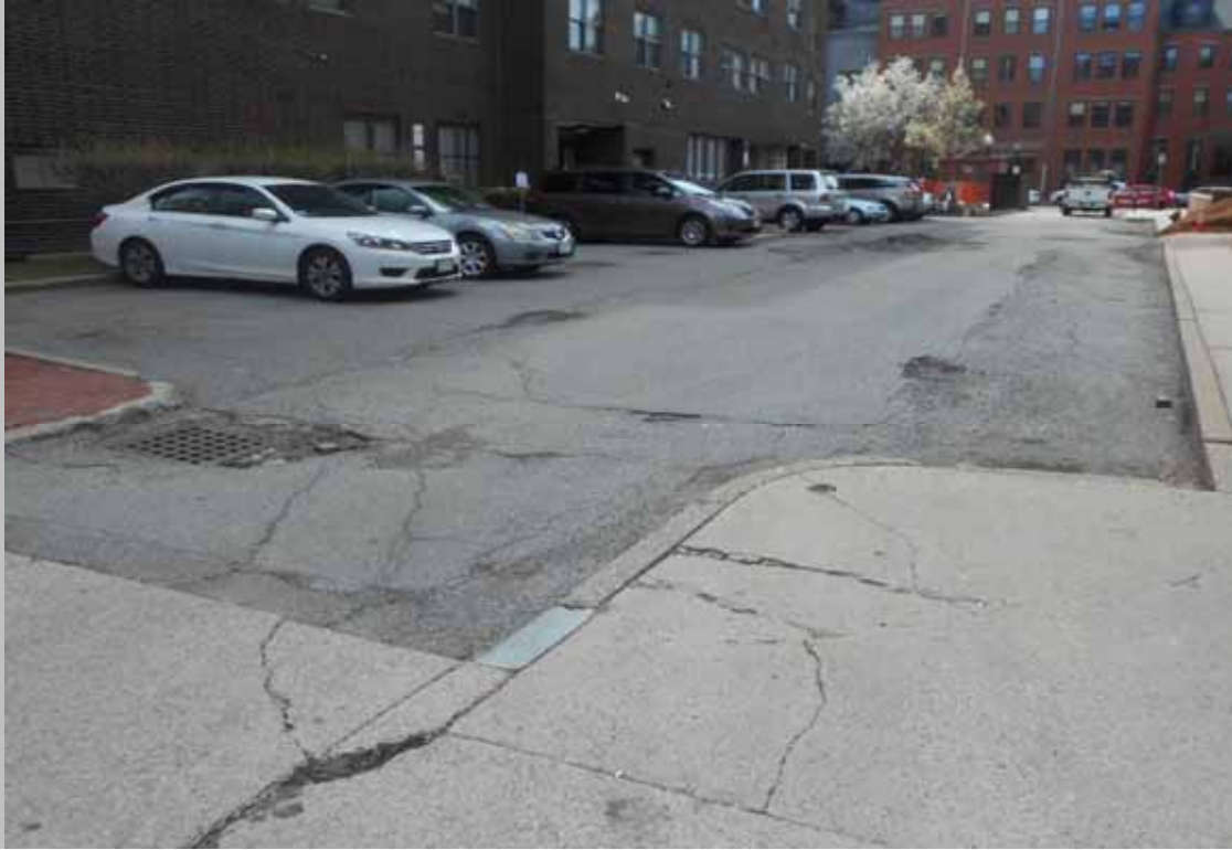
View of the parking lot in need of re-surfacing, re-sealing, and re-stripping (Non-Critical Repairs)
