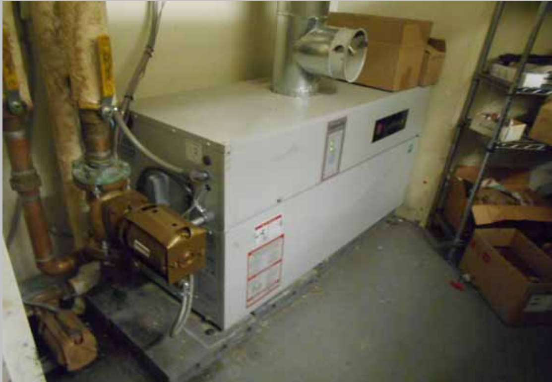
View of the DHW boiler
