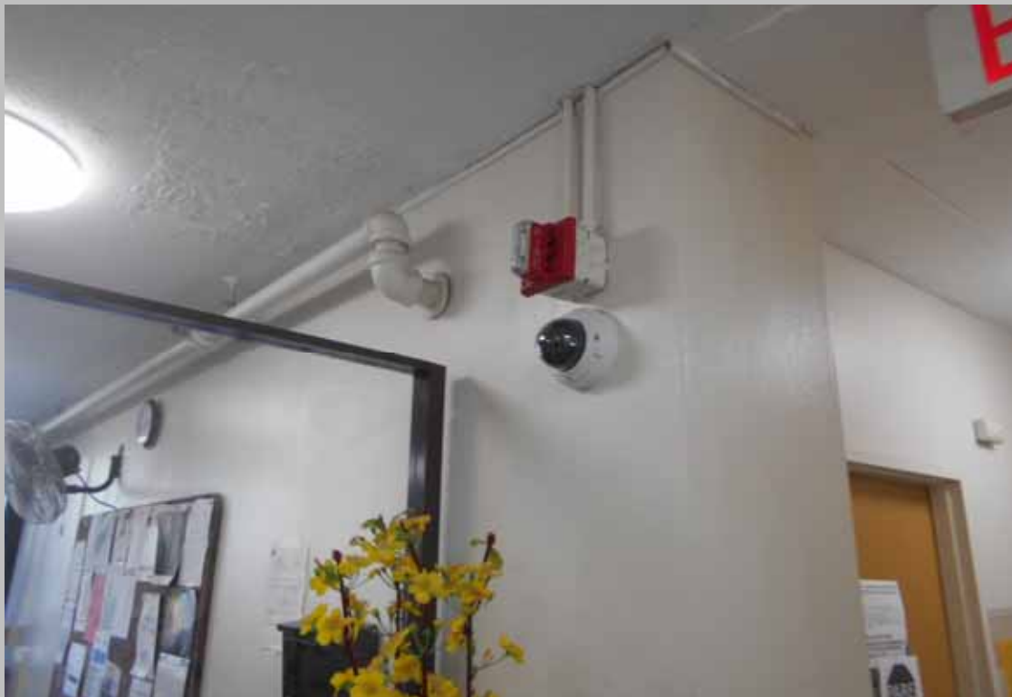
View of a fire alarm
