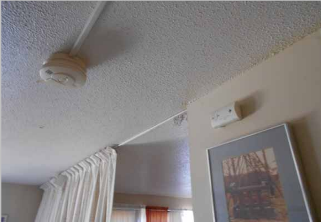
View of smoke detector and carbon monoxide detector – dwelling unit
