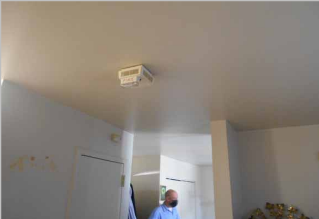
View of an A/V alarm – dwelling unit
