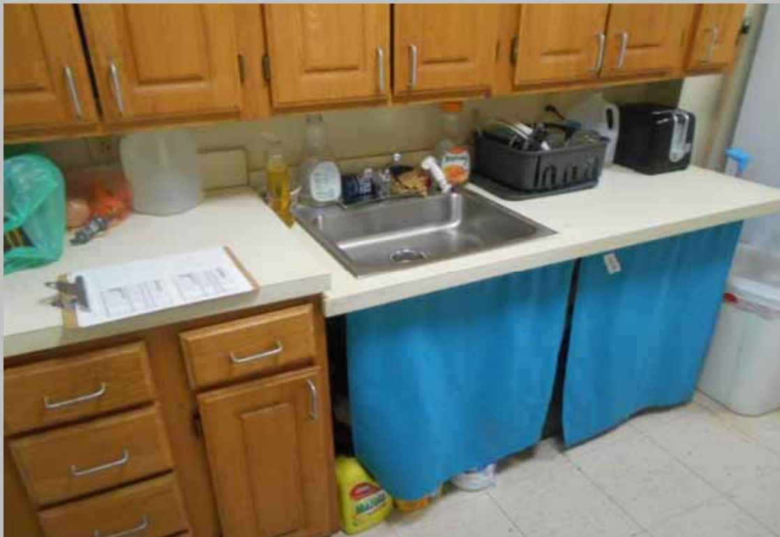
View of the roll-under sink within designated handicapped Unit 507 featuring levered hardware
