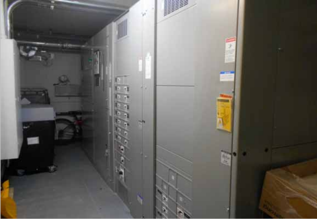
View of switchboard
