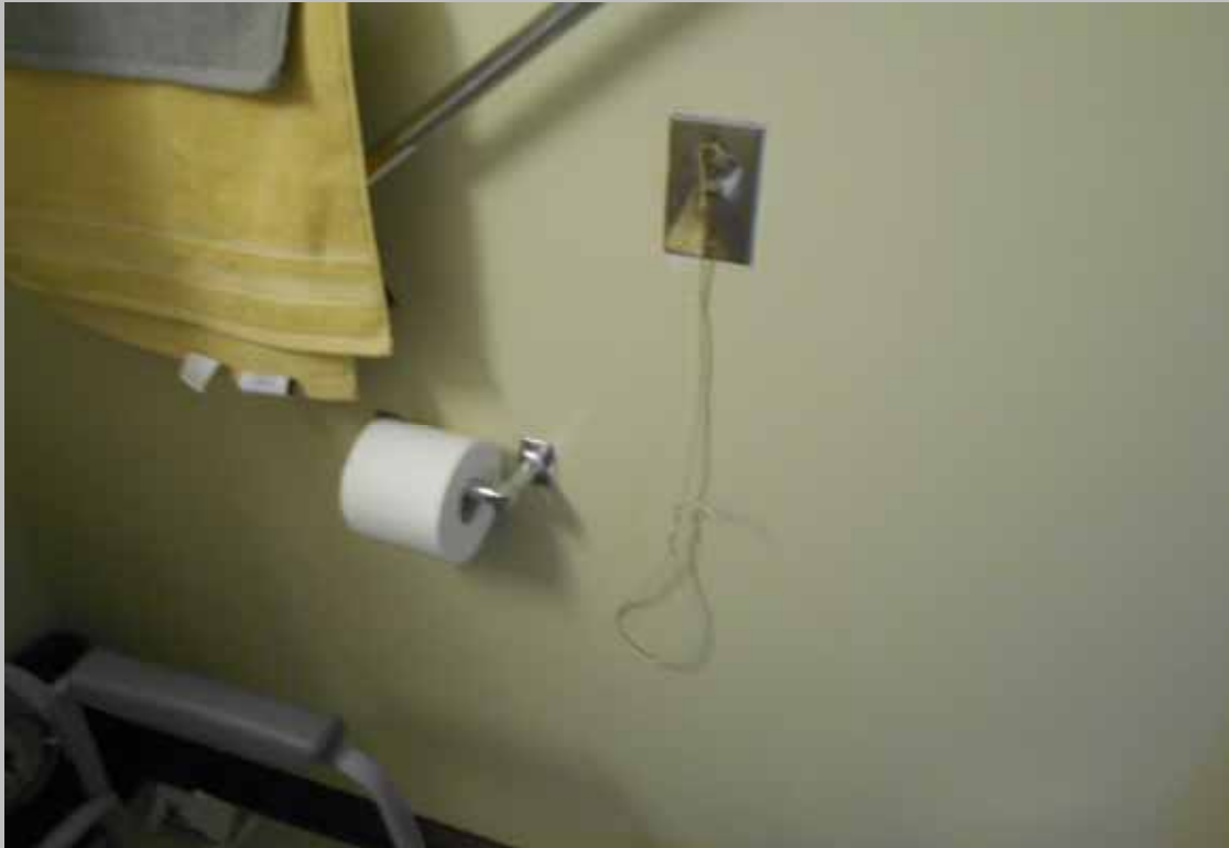
View of emergency pull cord – dwelling unit
