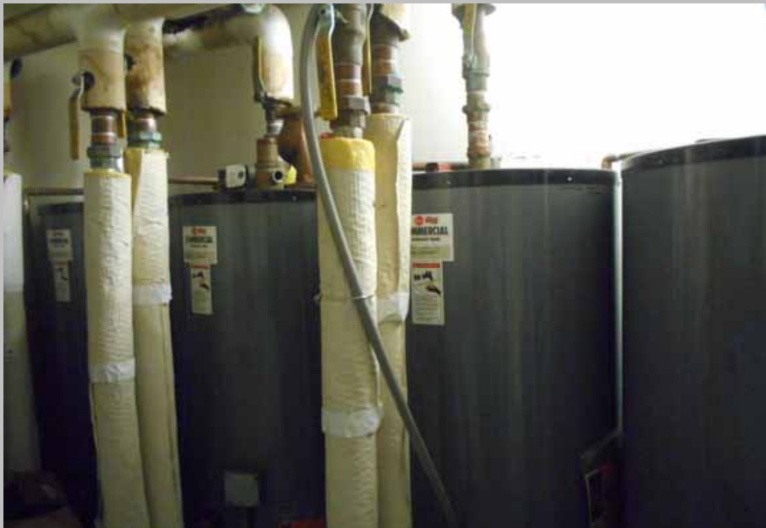
View of water storage tanks
