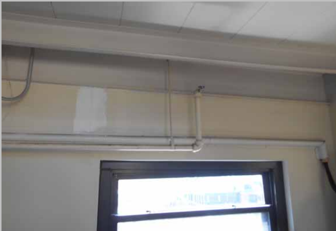
View of a sprinkler head
