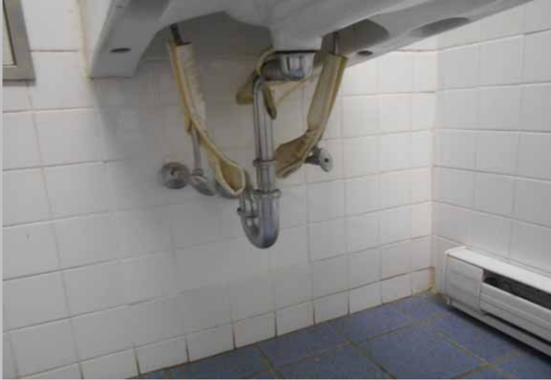
The Men's and Women's public restroom sinks feature non-compliant partial scald and abrasion protection at under-sink plumbing (Critical Repair)
