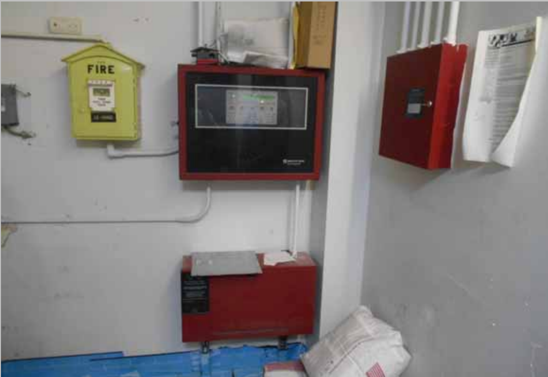
View of fire alarm control panel
