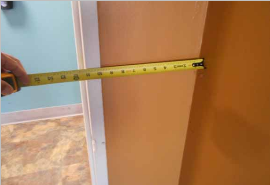
The common laundry room door does not feature 18 inches at the pull side of the door (Critical Repair)
