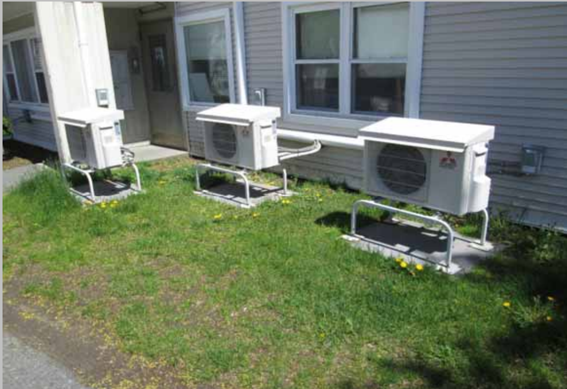
Mini-Split HVAC Units
