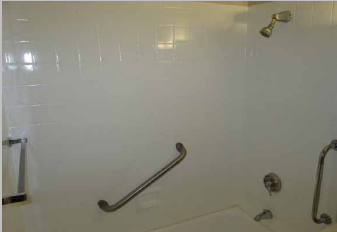
Shower/tub with tile surrounds
