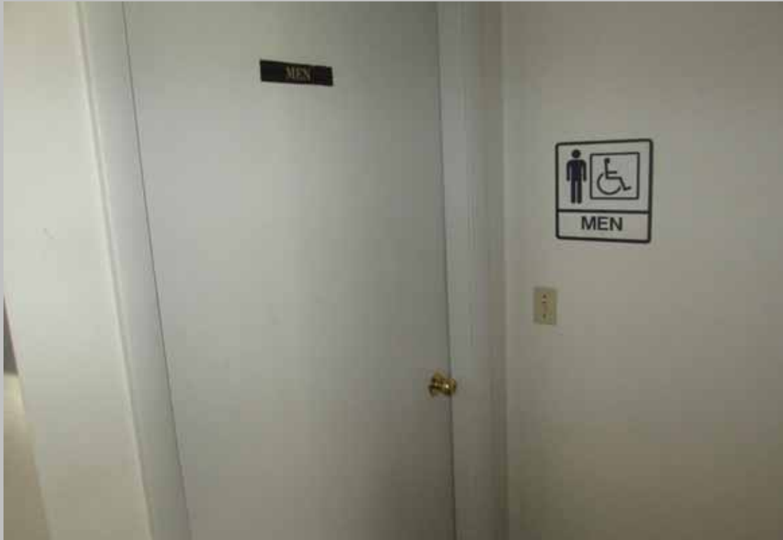
Men's public restroom with non-compliant door hardware (Critical-Repair)
