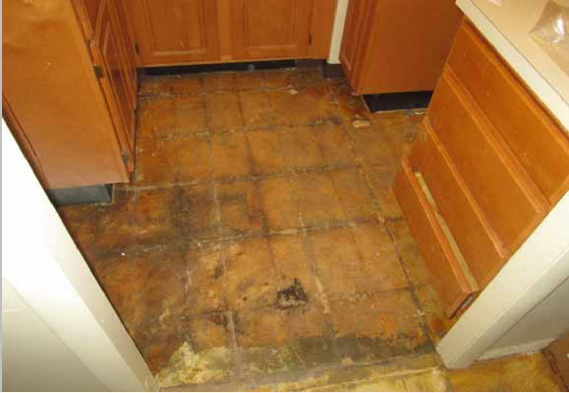
Down unit#16 (Non-Critical Repair)
