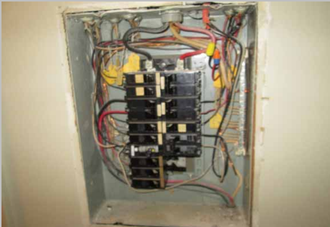
Typical dwelling unit electrical breaker panel
