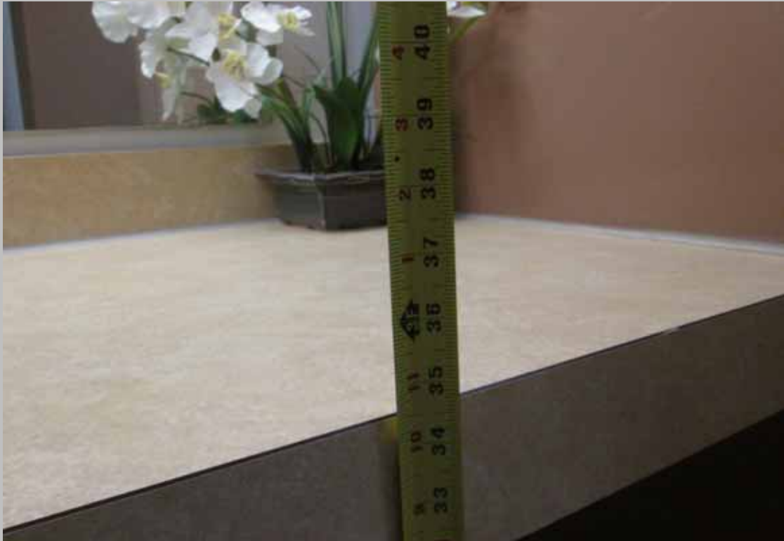
View of the women's public restroom sink mounted higher than 34-inches above the finished floor (Critical Repair)
