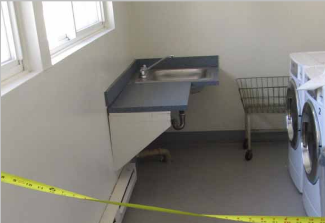
View of the common area laundry room sink lacking scald and abrasion protection (Critical Repair)
