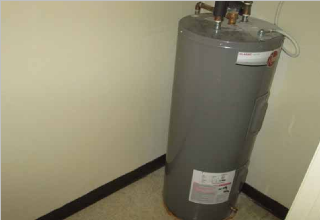
Typical dwelling unit electric water heater
