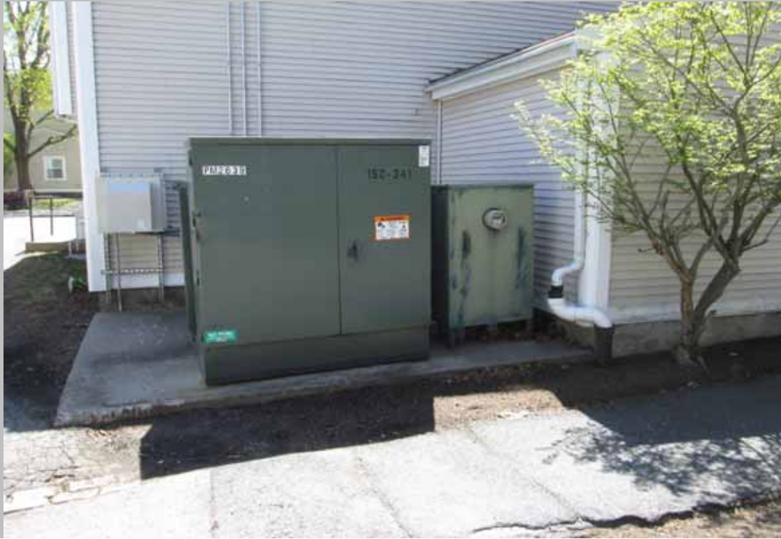
Pad mounted transformer
