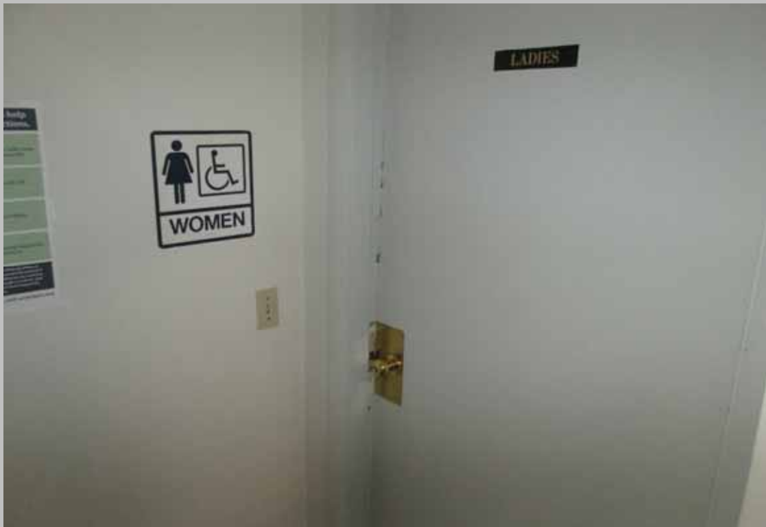
Women's public restroom with non-compliant door hardware (Critical-Repair)
