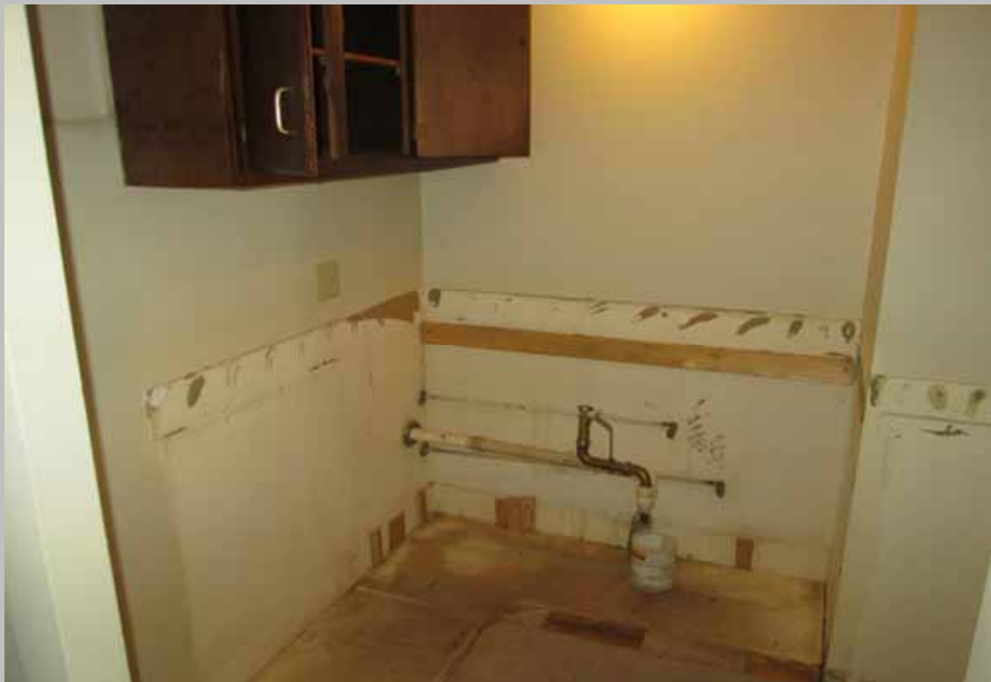
Down unit #98 (Non-Critical Repair)
