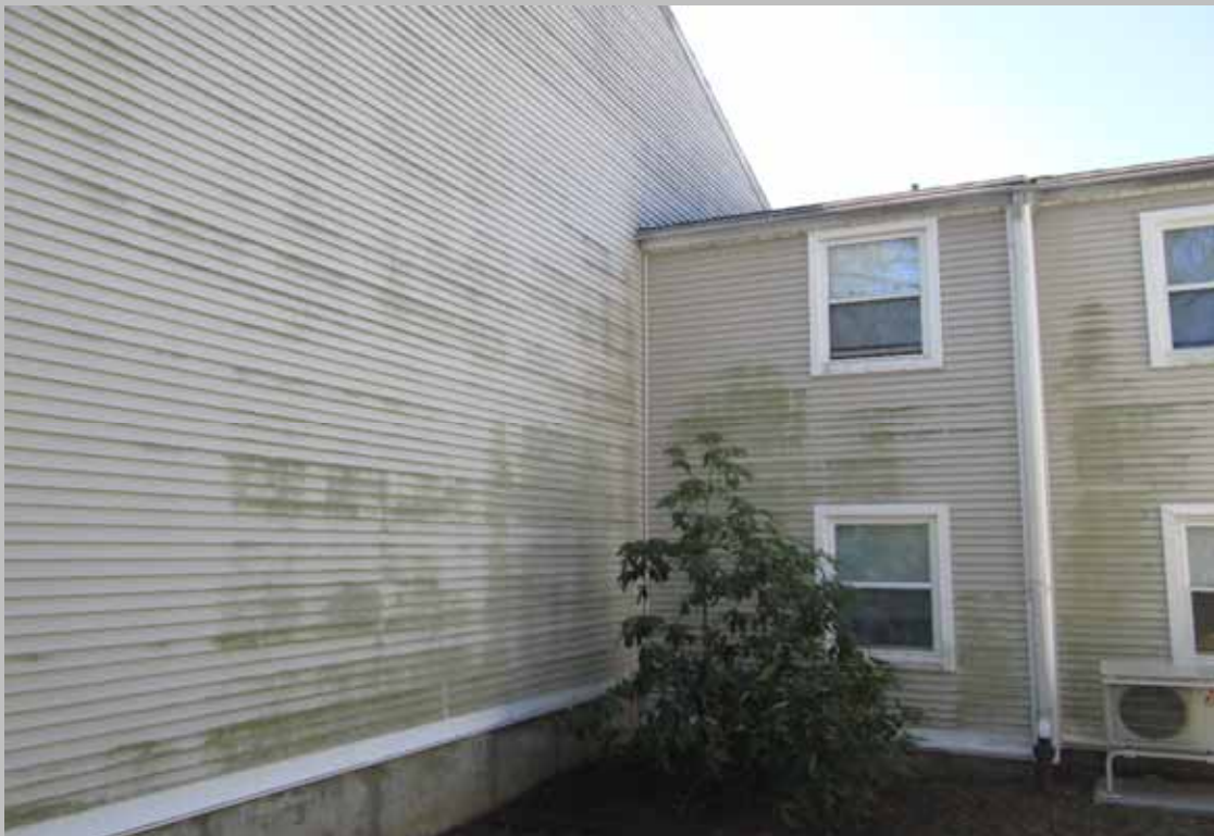
Mildew observed (Non-Critical Repair)
