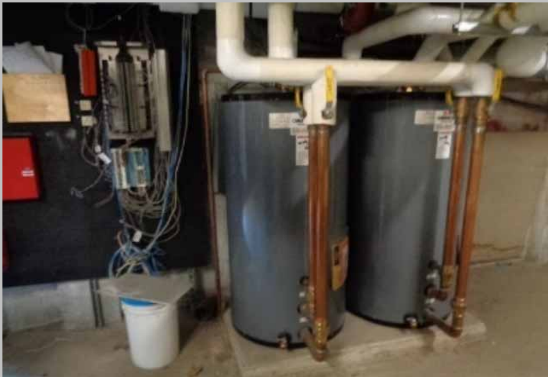
Central hot water heaters
