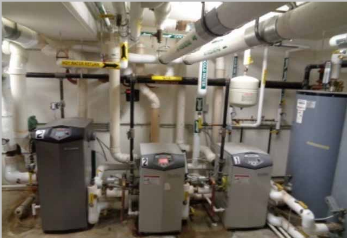
Site heating/DHW boiler equipment
