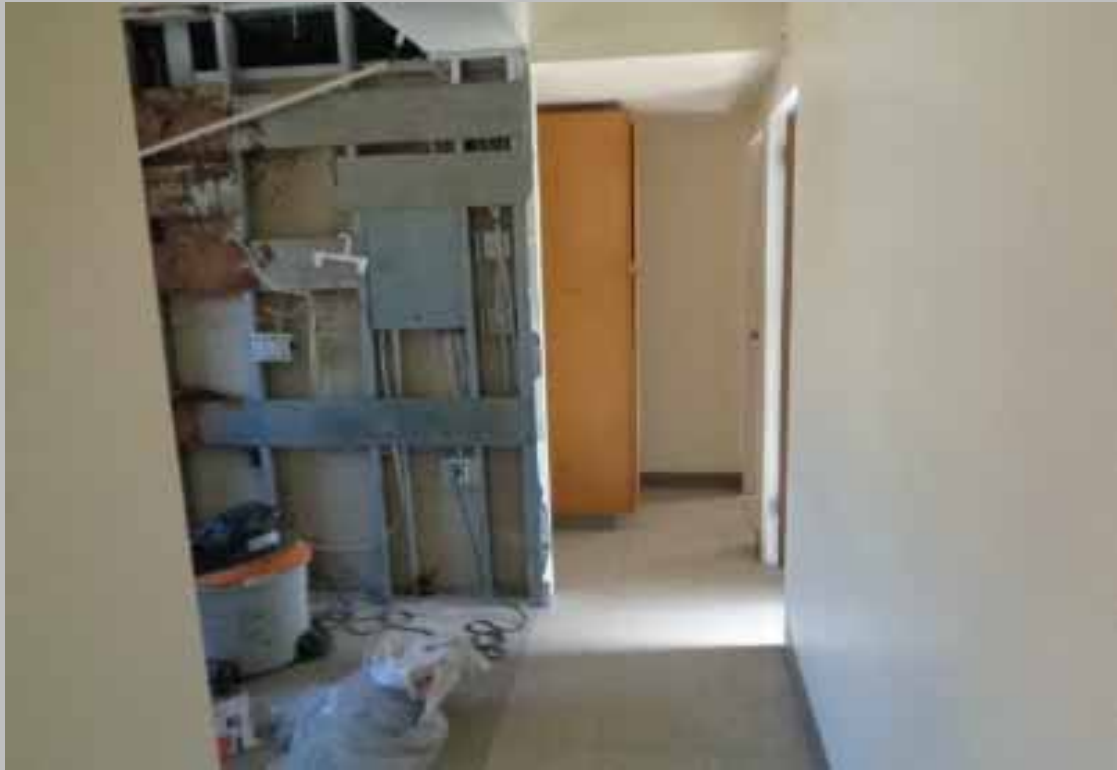
Down unit (Non-Critical Repair)
