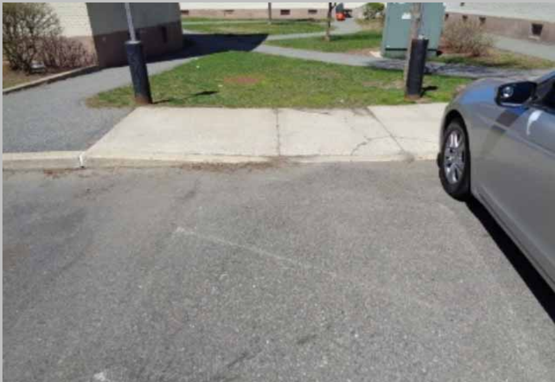
Faded line striping (Non-Critical Repair)
