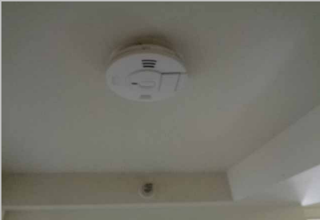
Dwelling unit smoke detector
