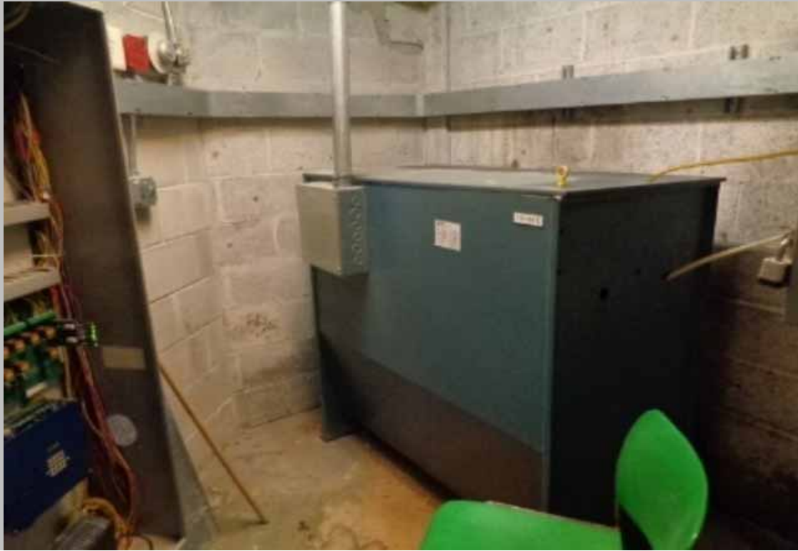
Hydraulic elevator equipment room
