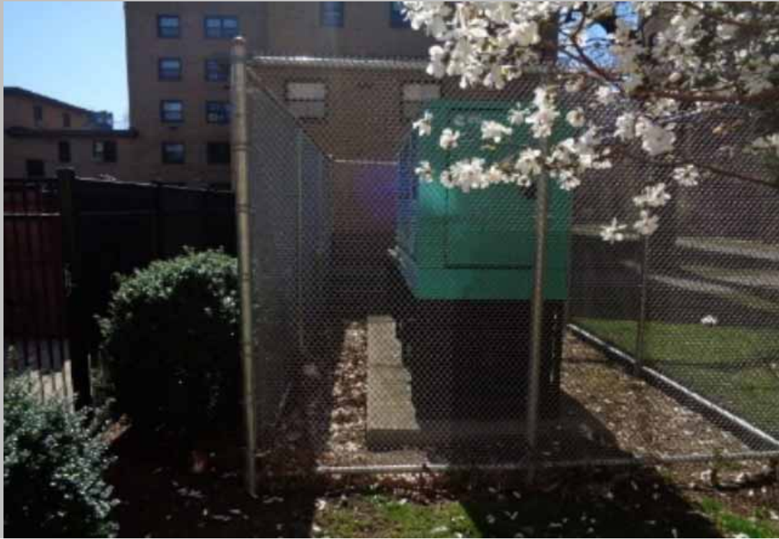
Typical Cummins Generator
