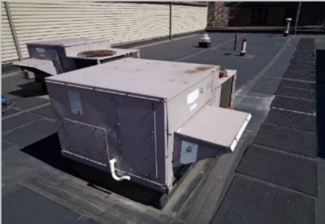
Roof-top HVAC package unit
