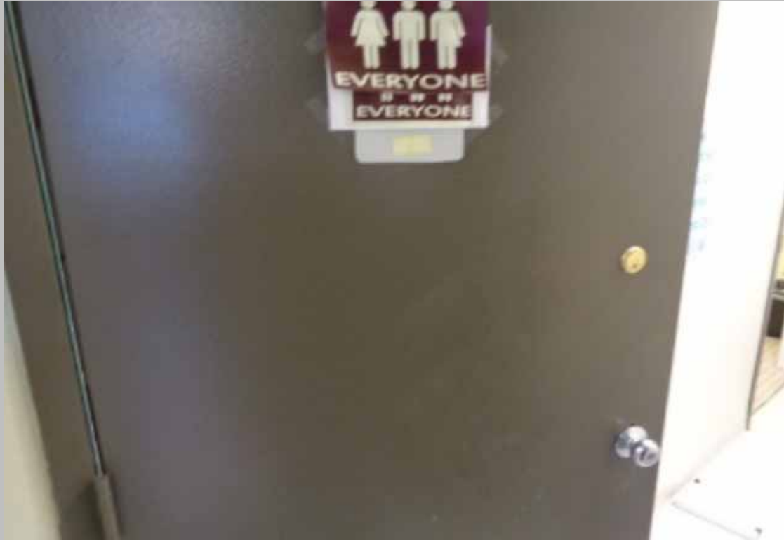
Common restroom door with non-compliant knob hardware (Critical Repair)
