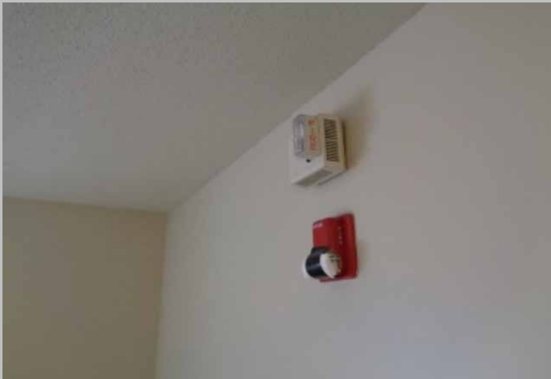
Handicapped unit fire safety
