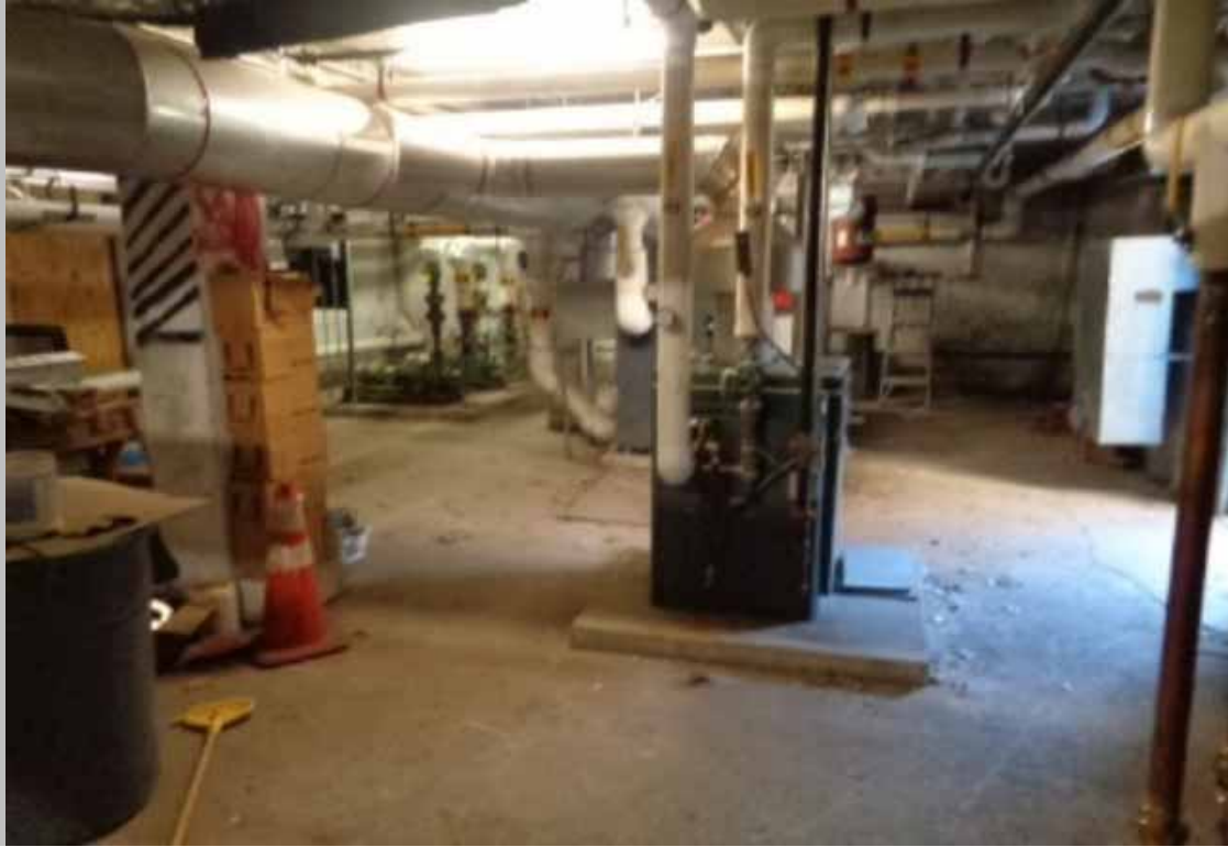
Typical mechanical basement area
