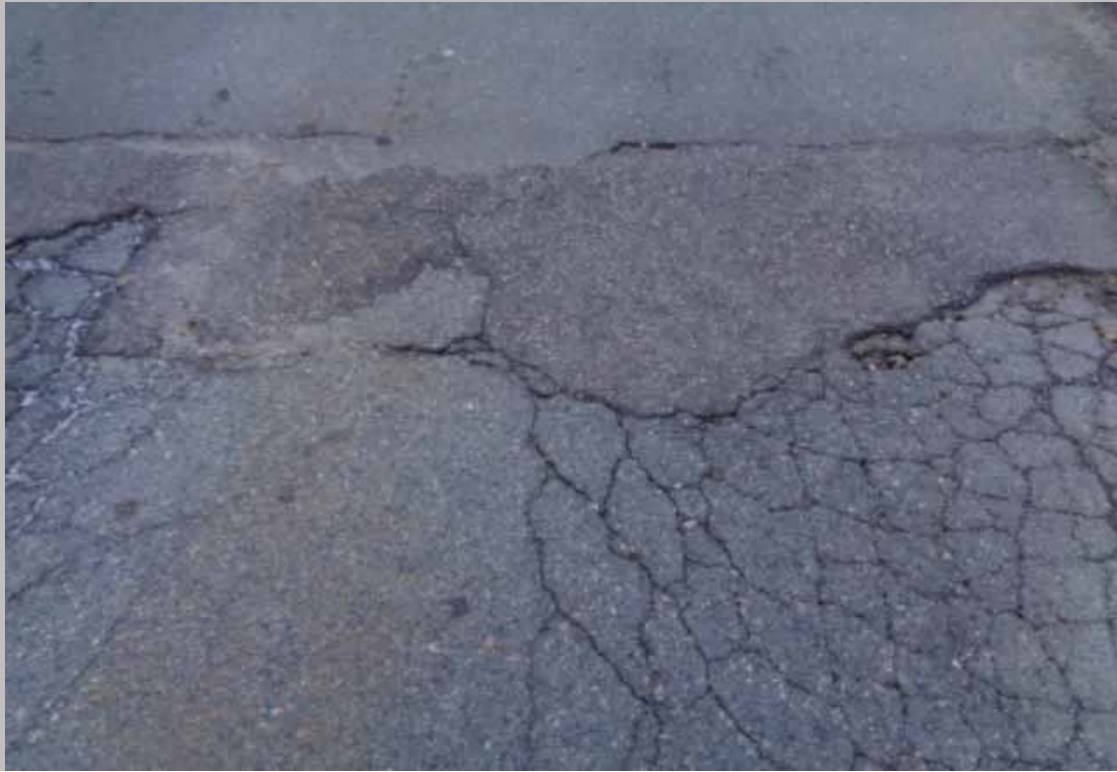
Asphalt parking area (Non-Critical Repair)
