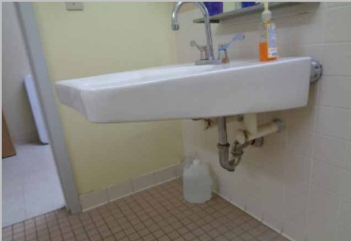
Common restroom missing S&A protection (Critical Repair)
