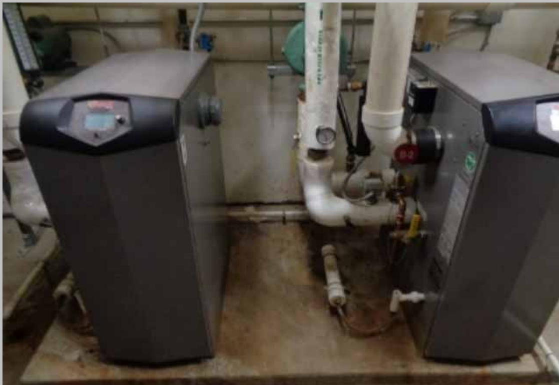
Site central boilers
