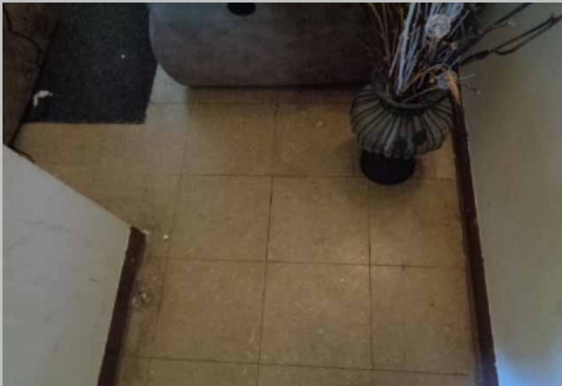
Unit flooring beyond EUL (Non-Critical Repair)
