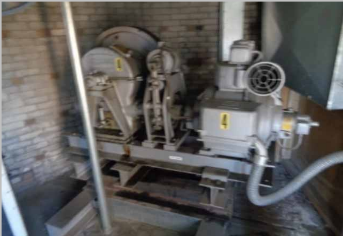
Typical hoist elevator equipment
