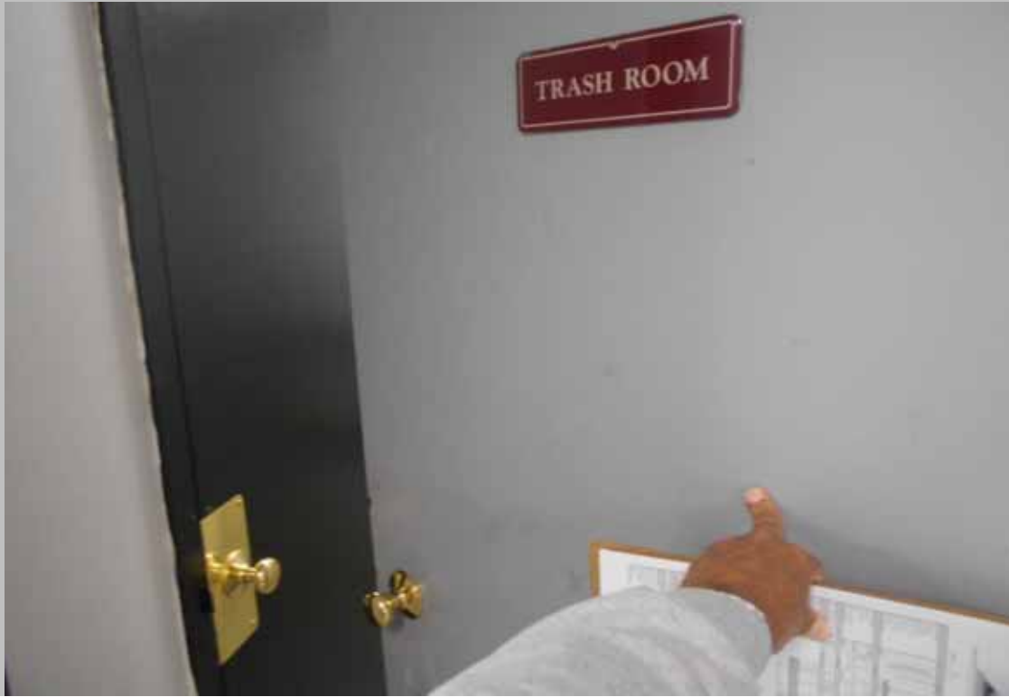
View of non-compliant knobbed hardware at a common area trash chute room entry door
