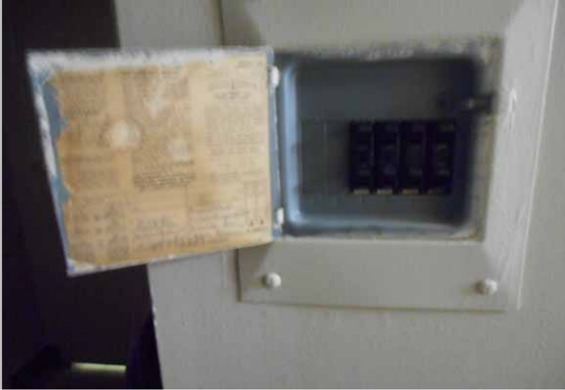
View of electric breaker panel - dwelling unit
