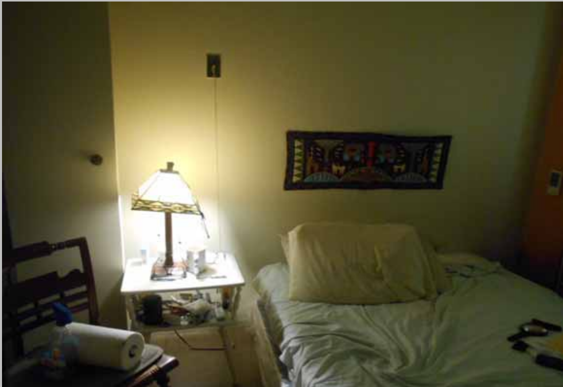
View of emergency pull cord - dwelling unit
