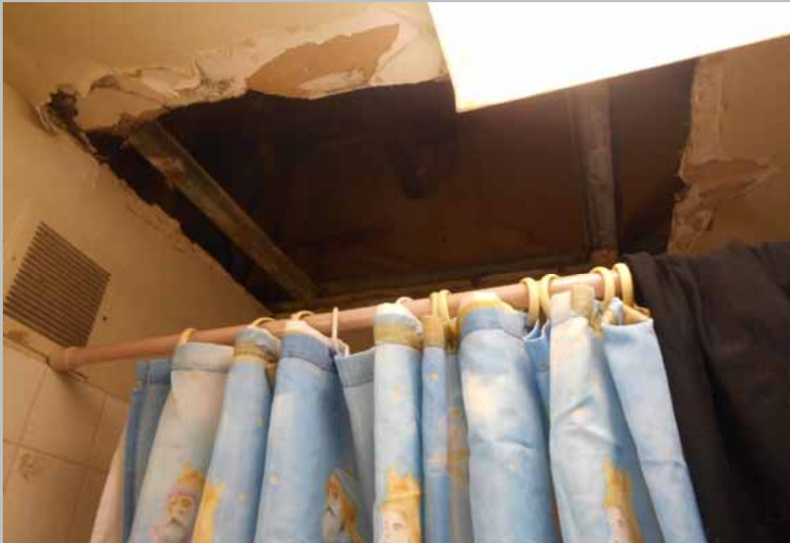
View of damaged GWB in the bathroom of dwelling unit 503 (Non-Critical Repair)
