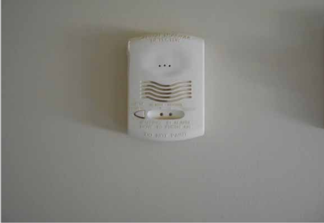
View of carbon monoxide detector – dwelling unit
