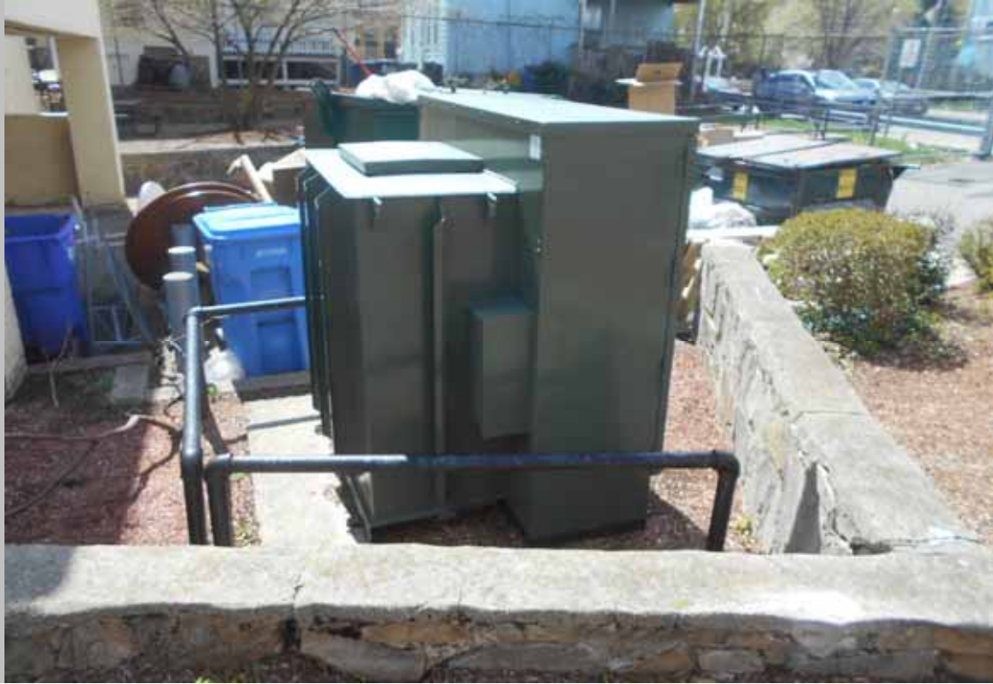
View of pad mounted electrical transformer
