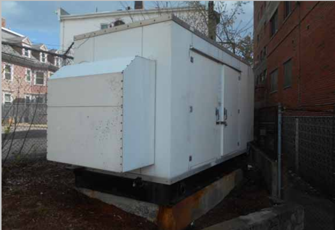
View of the property generator
