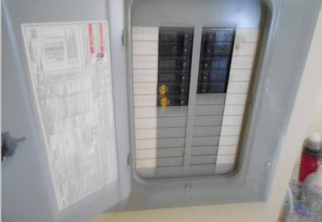
View of electric breaker panel – dwelling unit
