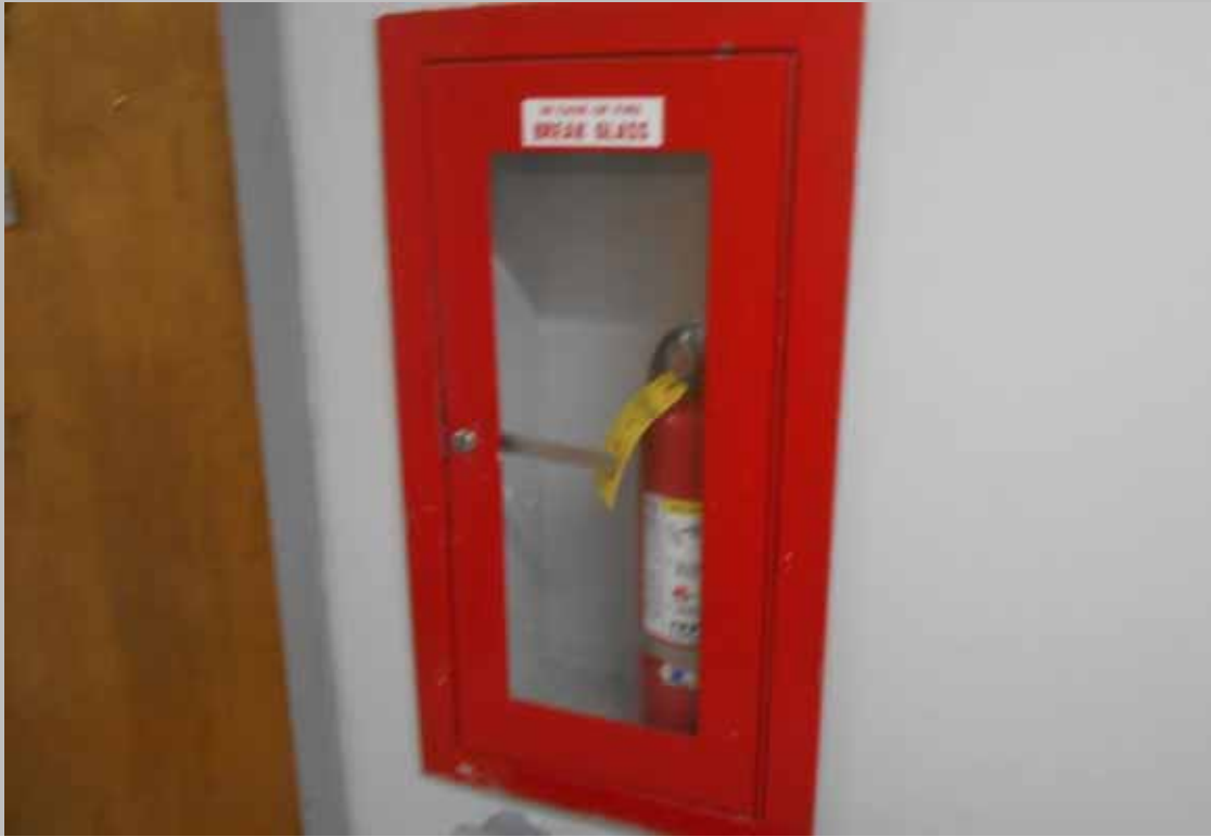
View of a fire extinguisher
