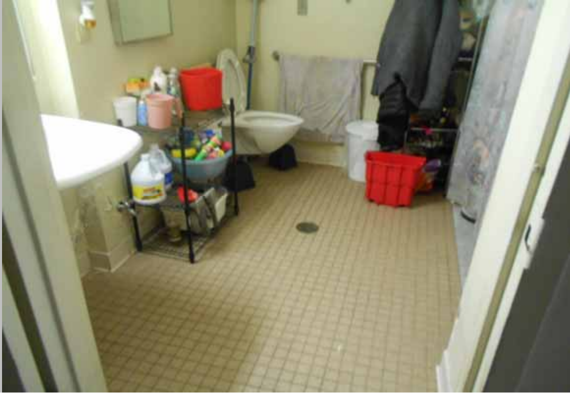
View of the bathroom within designated handicapped unit 411 – featuring compliant clear floor space at the fixtures, a roll-in shower, and roll-under access at the sink
