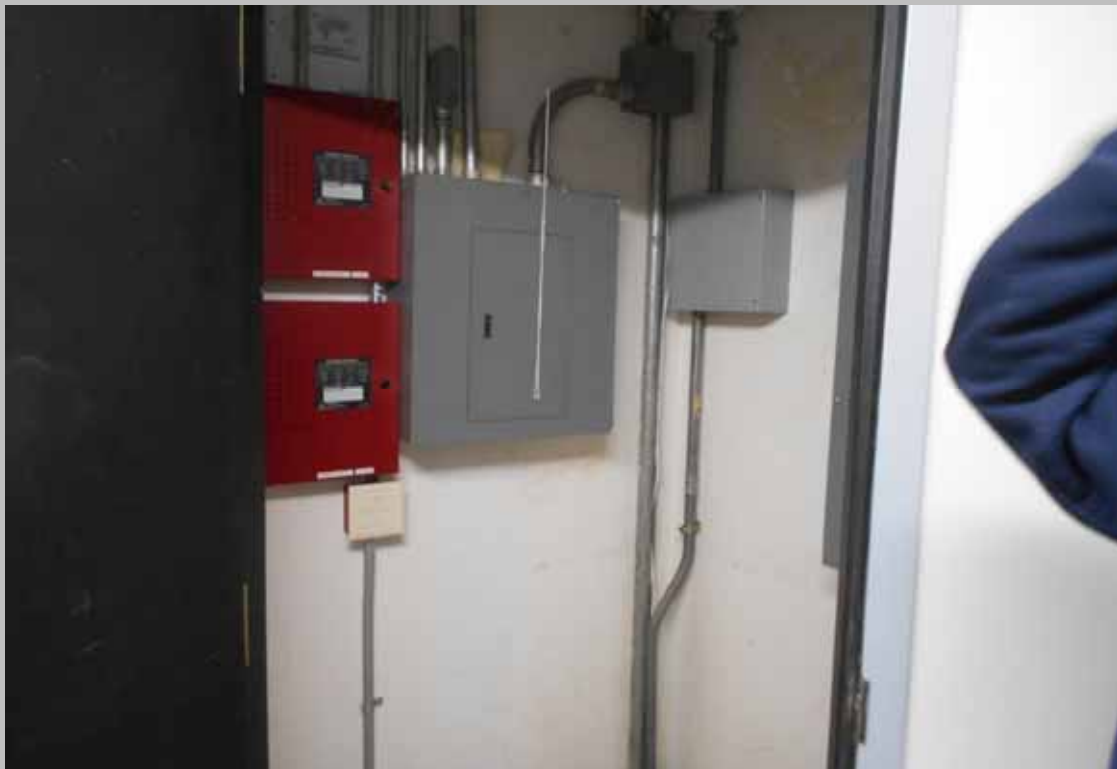
View of fire alarm control panel
