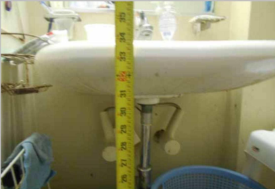
View of a compliant height bathroom sink within a designated handicapped dwelling unit lacking compliant scald and abrasion protection (Critical Repair)
