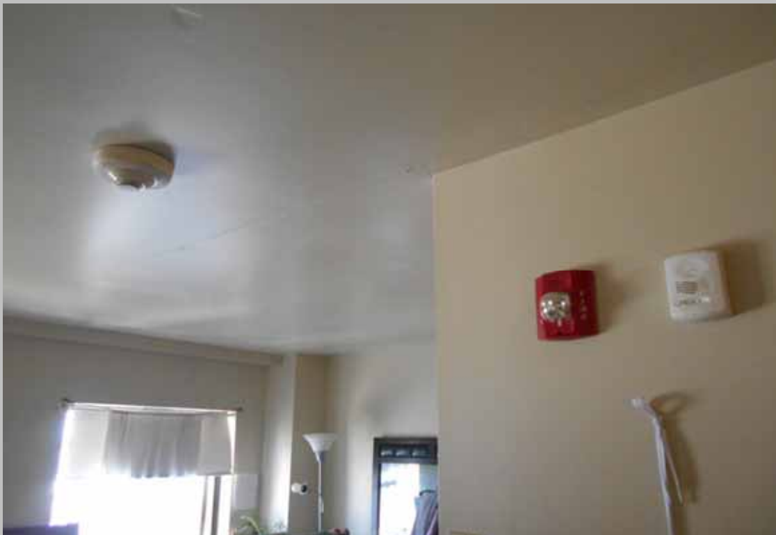
View of smoke detectors and fire alarm – dwelling unit
