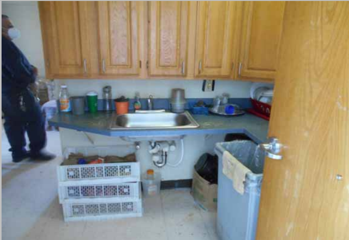
View of kitchen within designated handicapped unit 411 – featuring roll-under access and levered handle hardware
