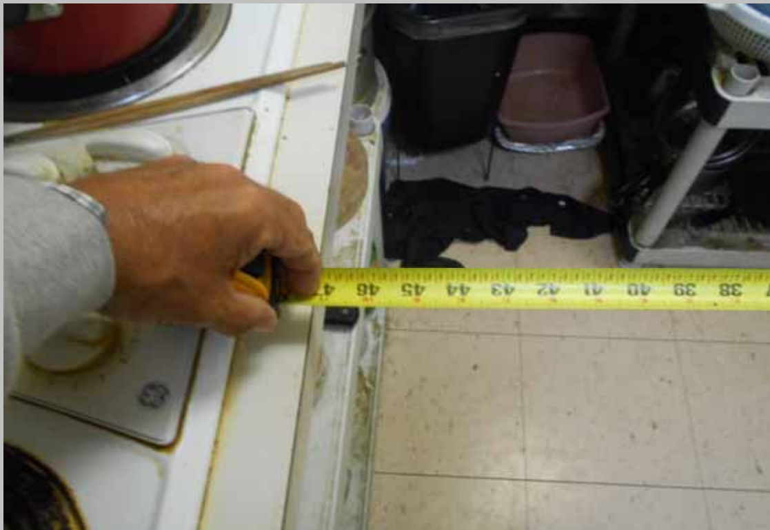
View of the kitchen within designated handicapped dwelling unit 611 lacking compliant clear floor space in the U-shaped kitchen
