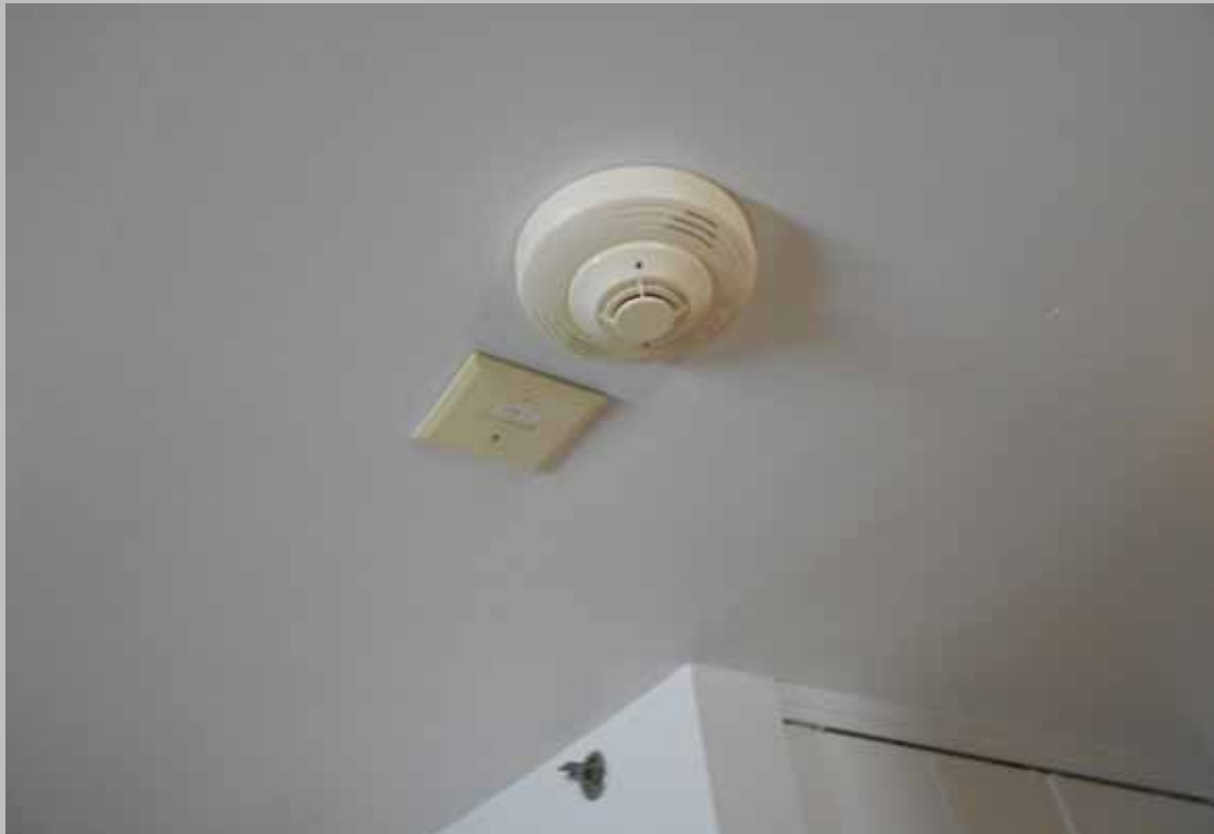
View of smoke detector – dwelling unit
