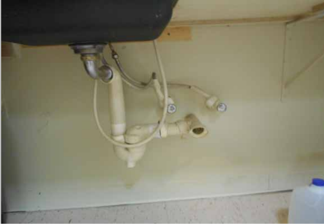
View of a compliant kitchen sink within a designated handicapped dwelling unit lacking compliant scald and abrasion protection (Critical Repair)
