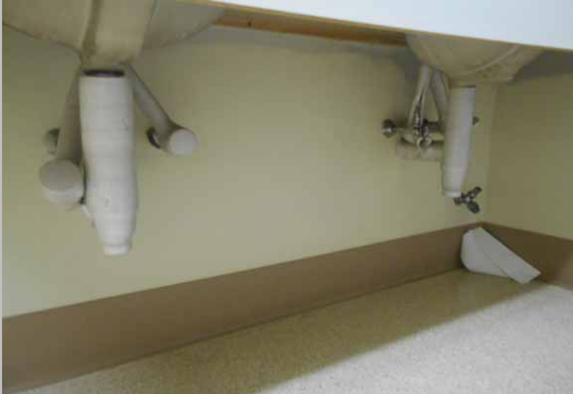
View of non-compliant partial scald and abrasion protection at the women's public restroom (Critical Repair)
