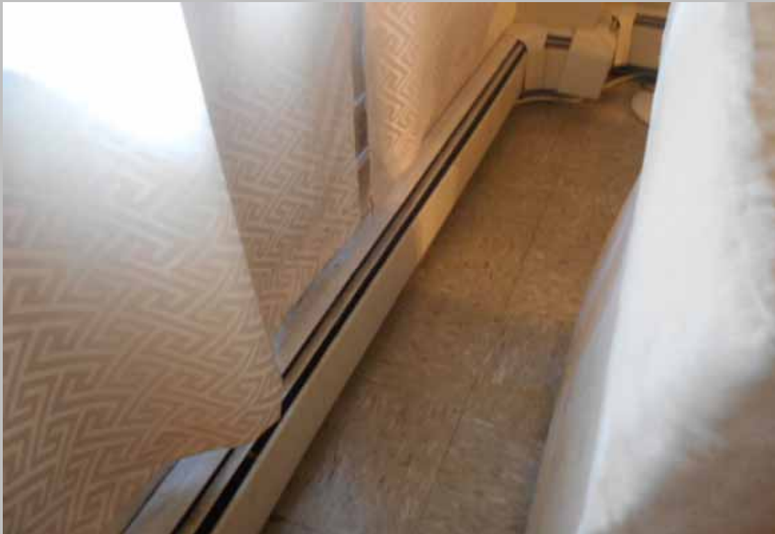
View of a baseboard heater – dwelling unit
