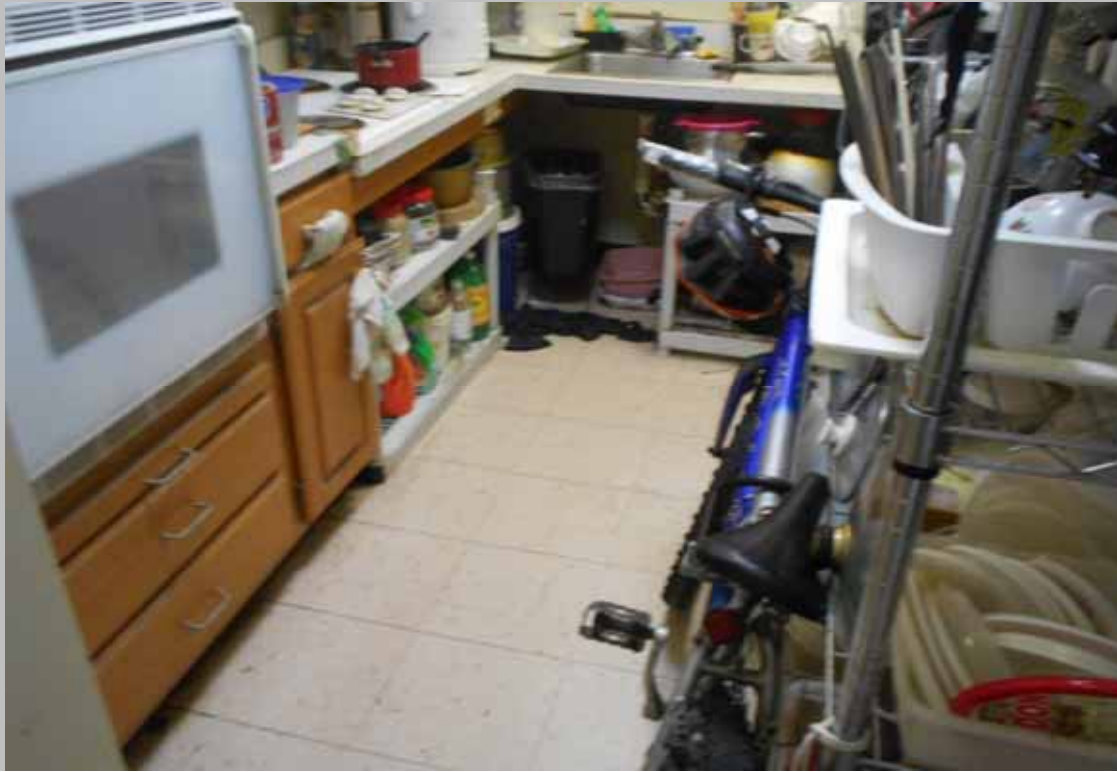
View of the kitchen within designated handicapped dwelling unit 611 lacking compliant clear floor space in the U-shaped kitchen
