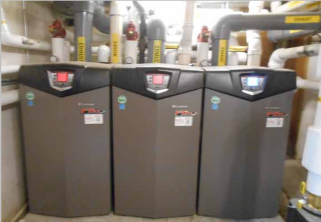
View of the property boilers
