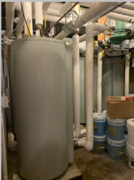
Hot water storage tank
