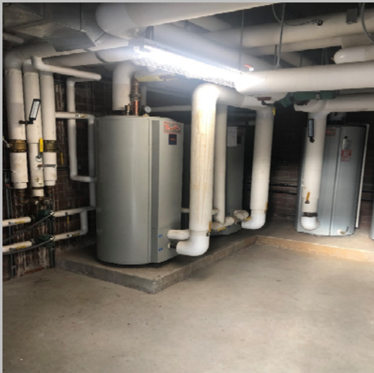
Hot water storage tanks
