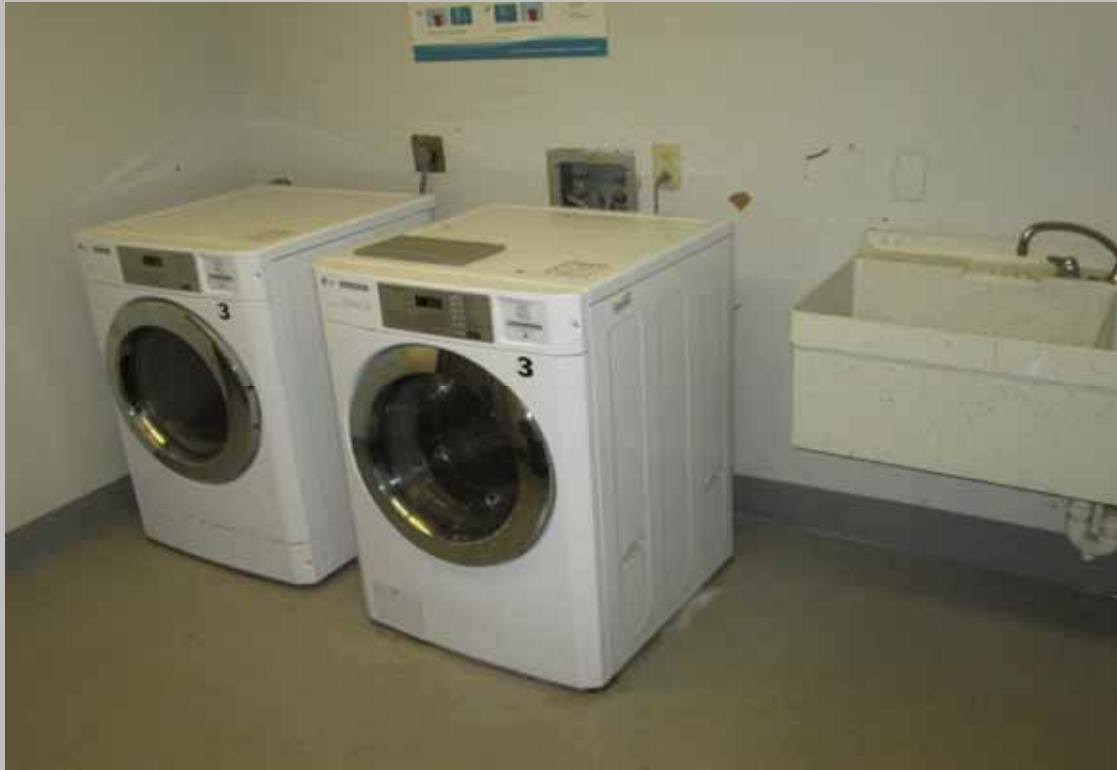
Typical laundry room
