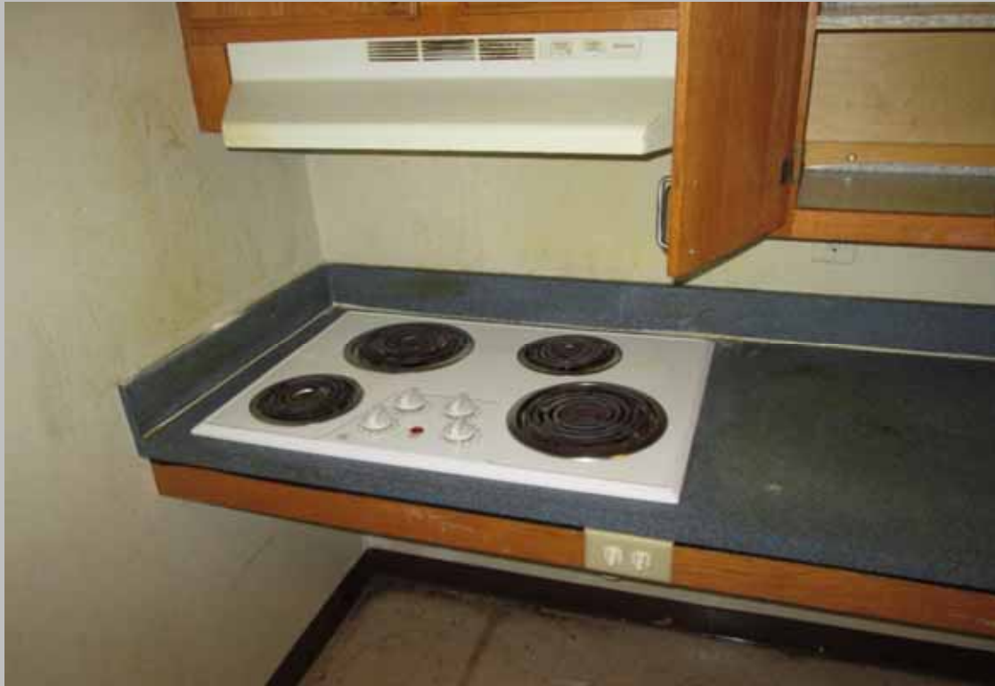
Designated handicapped unit electric cooktop
