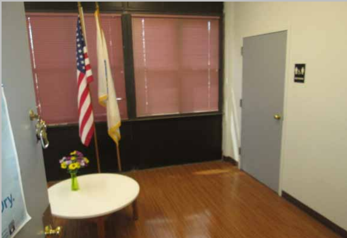
Community room area door and community uni-sex restroom door with non-compliant (knobbed) hardware (Critical Repair)
