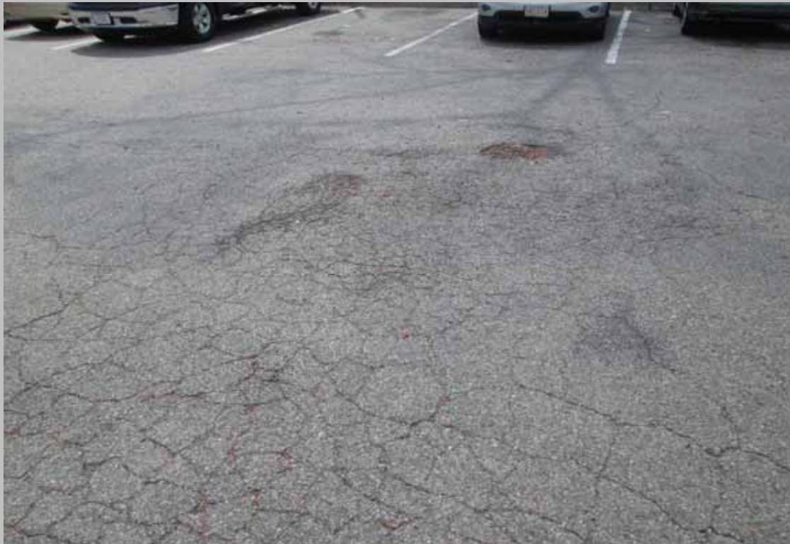
Site asphalt parking area (Non-Critical Repair)
