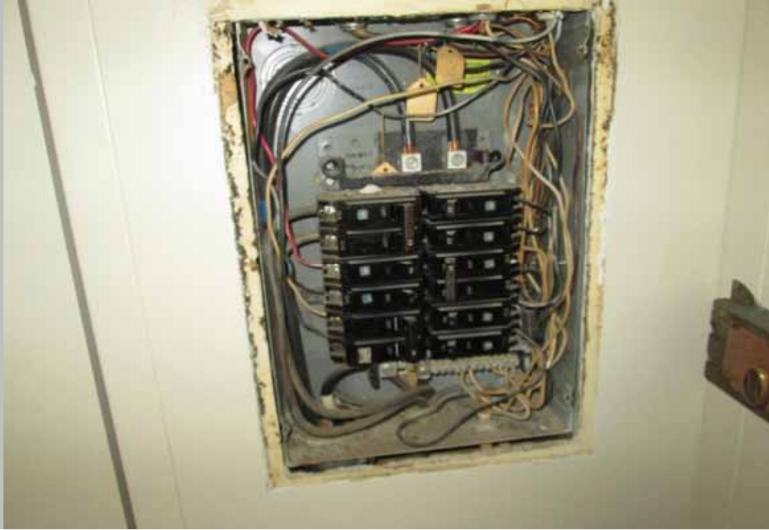
Typical building copper wiring/breaker panel view
