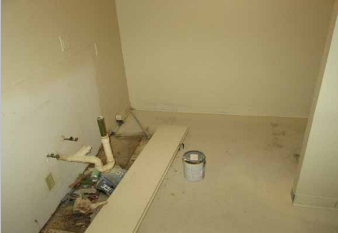
"Down" Unit 108 (Critical Repair)
