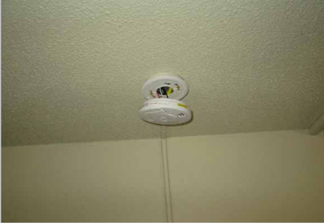
Hardwired smoke detectors outside of the sleeping area
