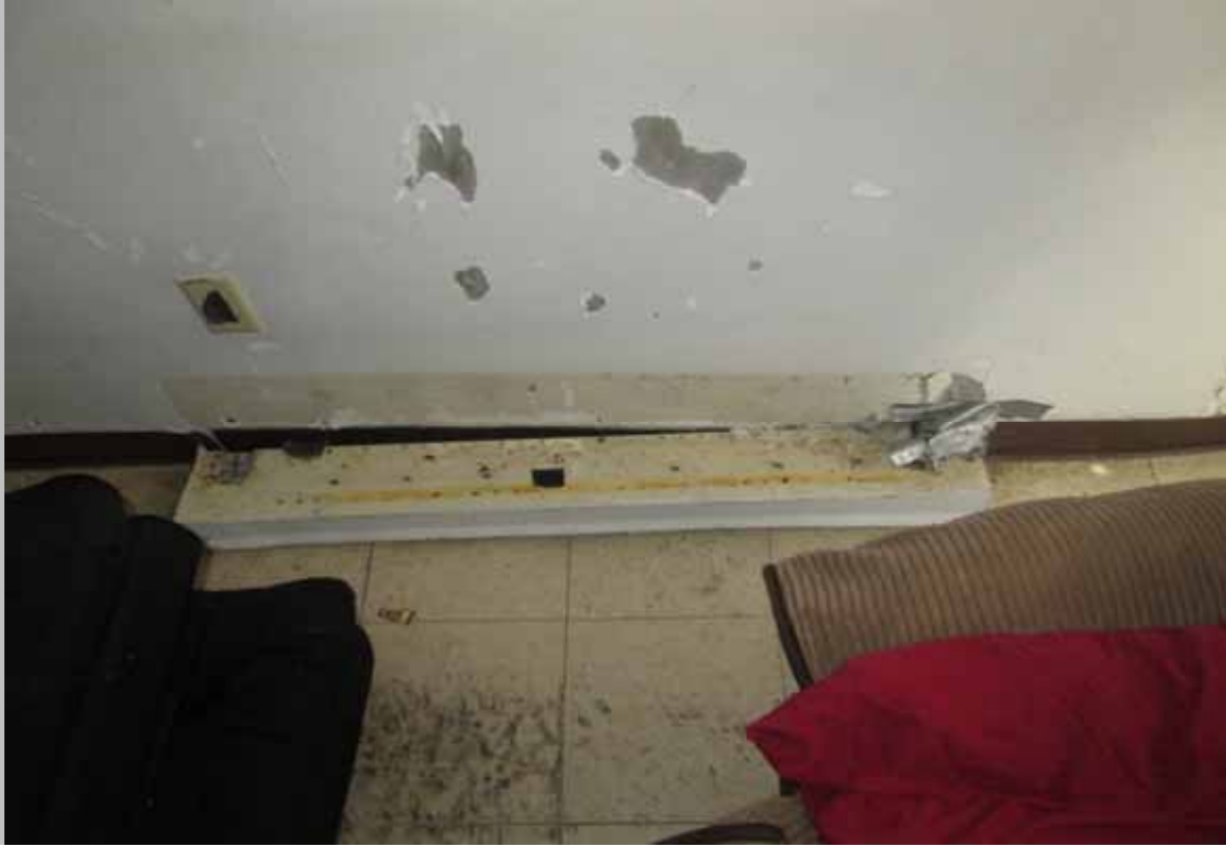
Damaged baseboard heater in Unit 318 (Non-Critical Repair)
