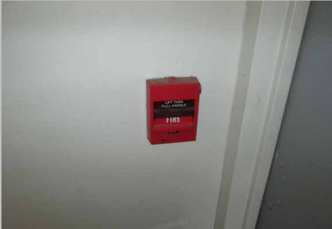
Common fire alarm
