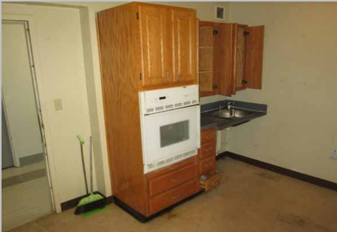
Designated handicapped unit wall-mounted oven
