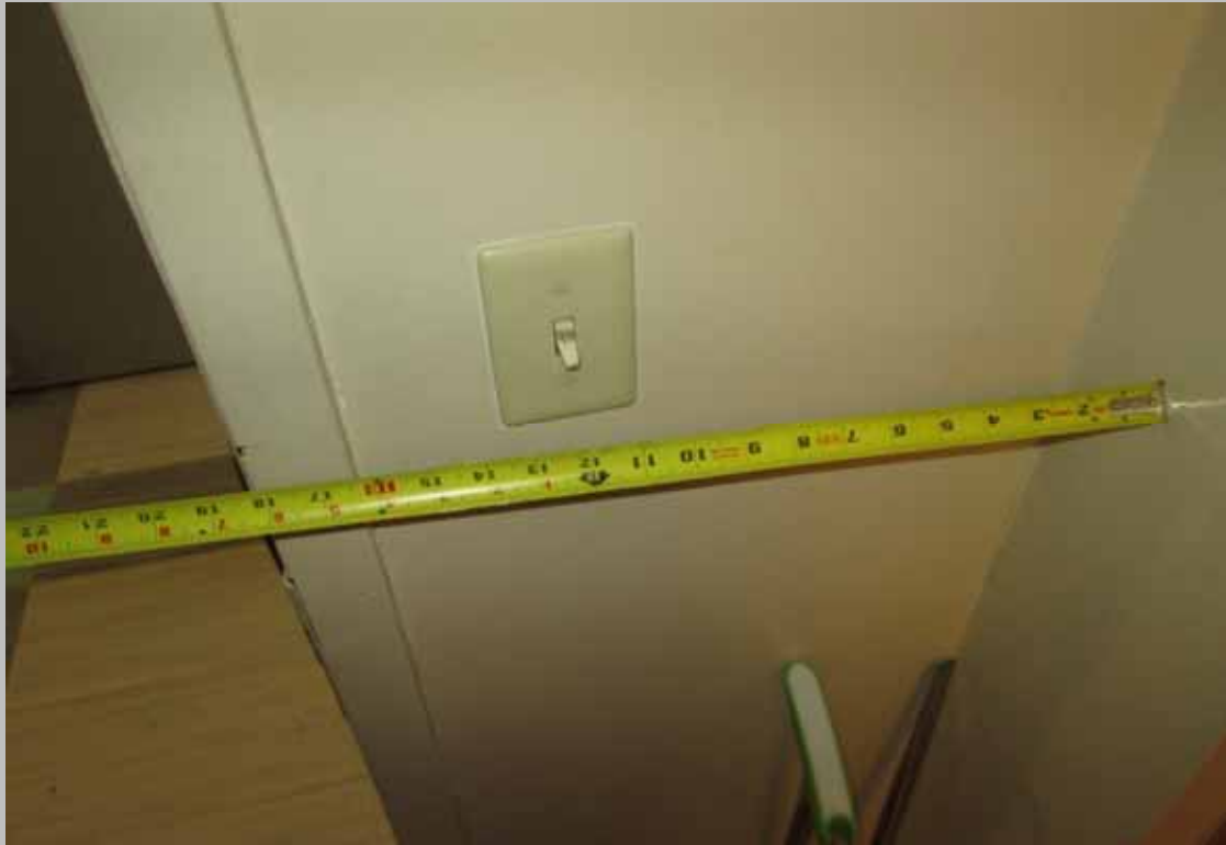
Compliant 18-inches at entry door
