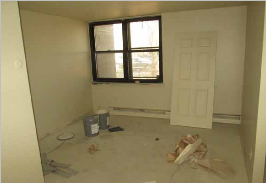
"Down" Unit 108 (Critical Repair)
