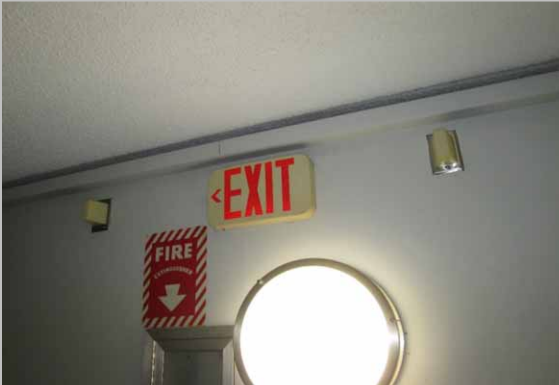
Common area fire safety/exit
