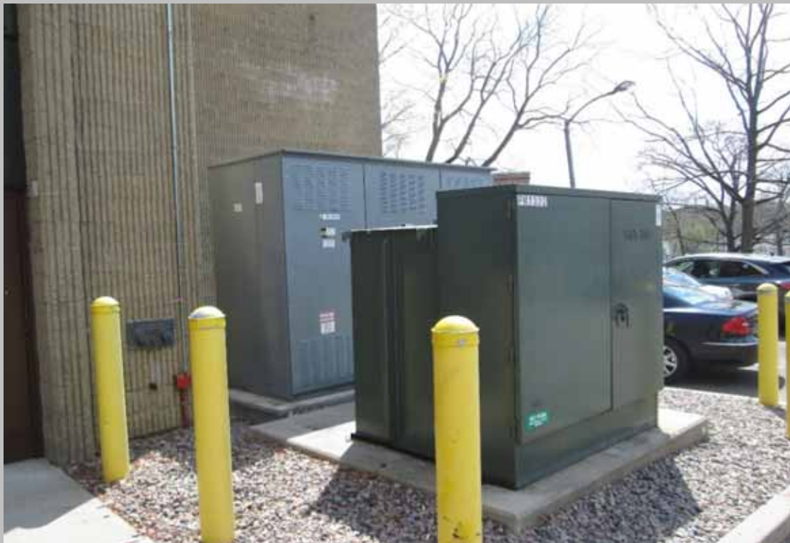
Pad mounted transformer
