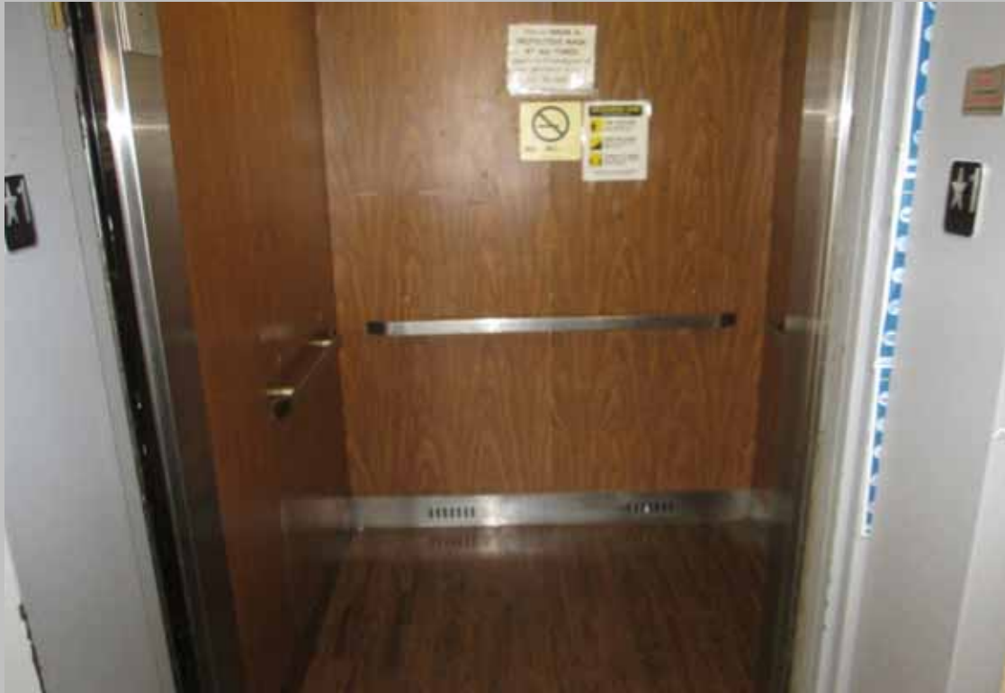
Typical elevator cab
