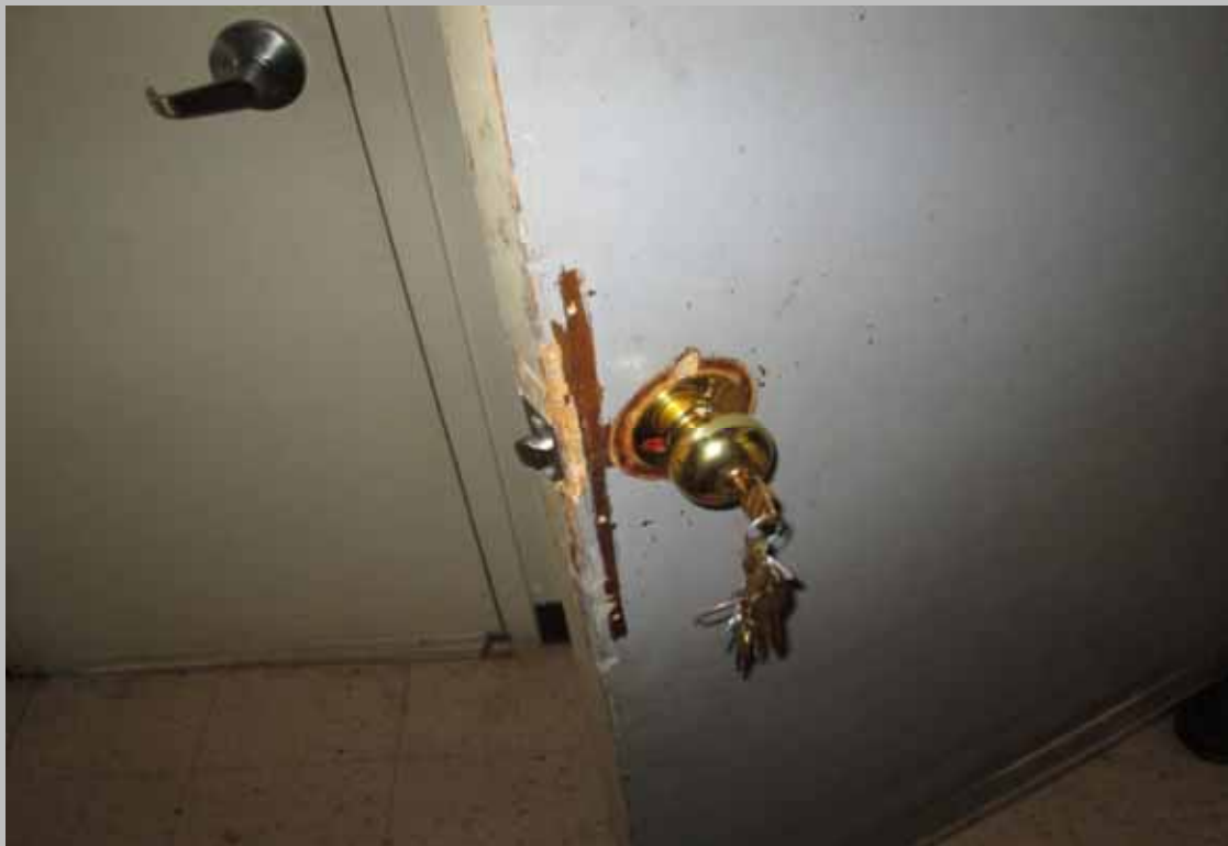
Handicapped Unit# 323 non-compliant door hardware (Critical Repair)
