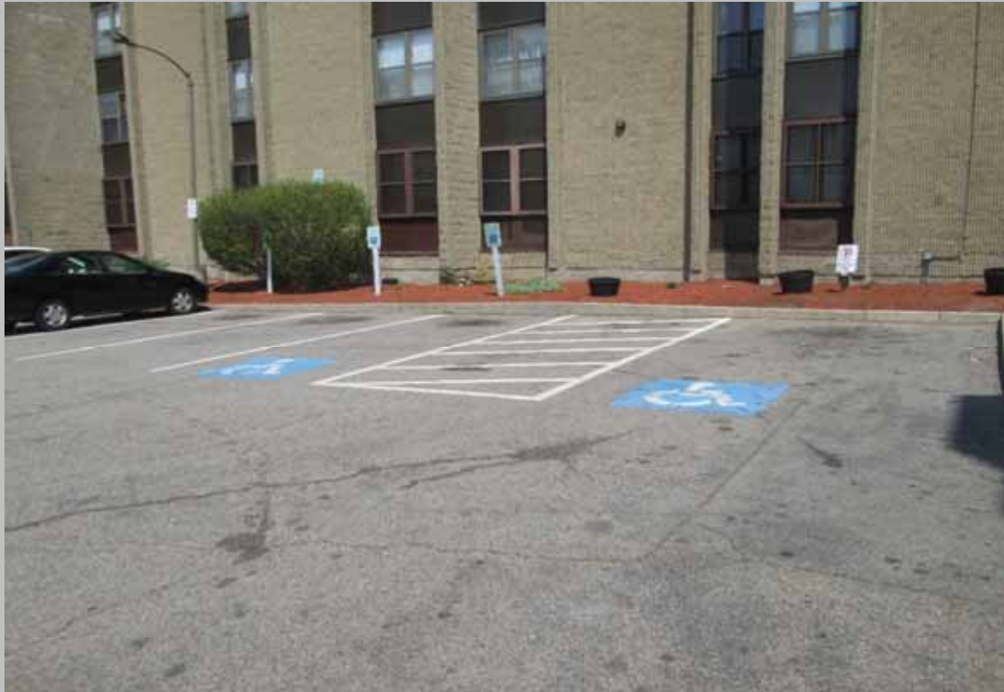
Handicapped parking without "Van-Accessible" sign (Critical Repair)
