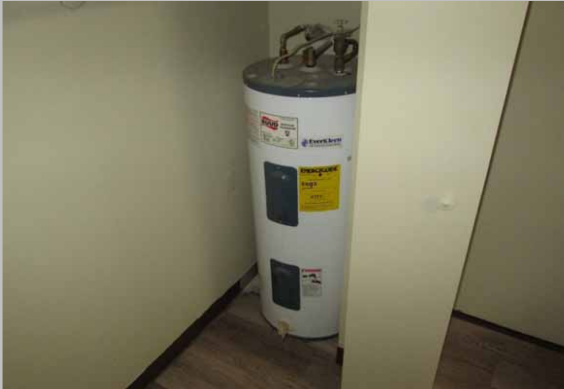
Dwelling unit hot water heater
