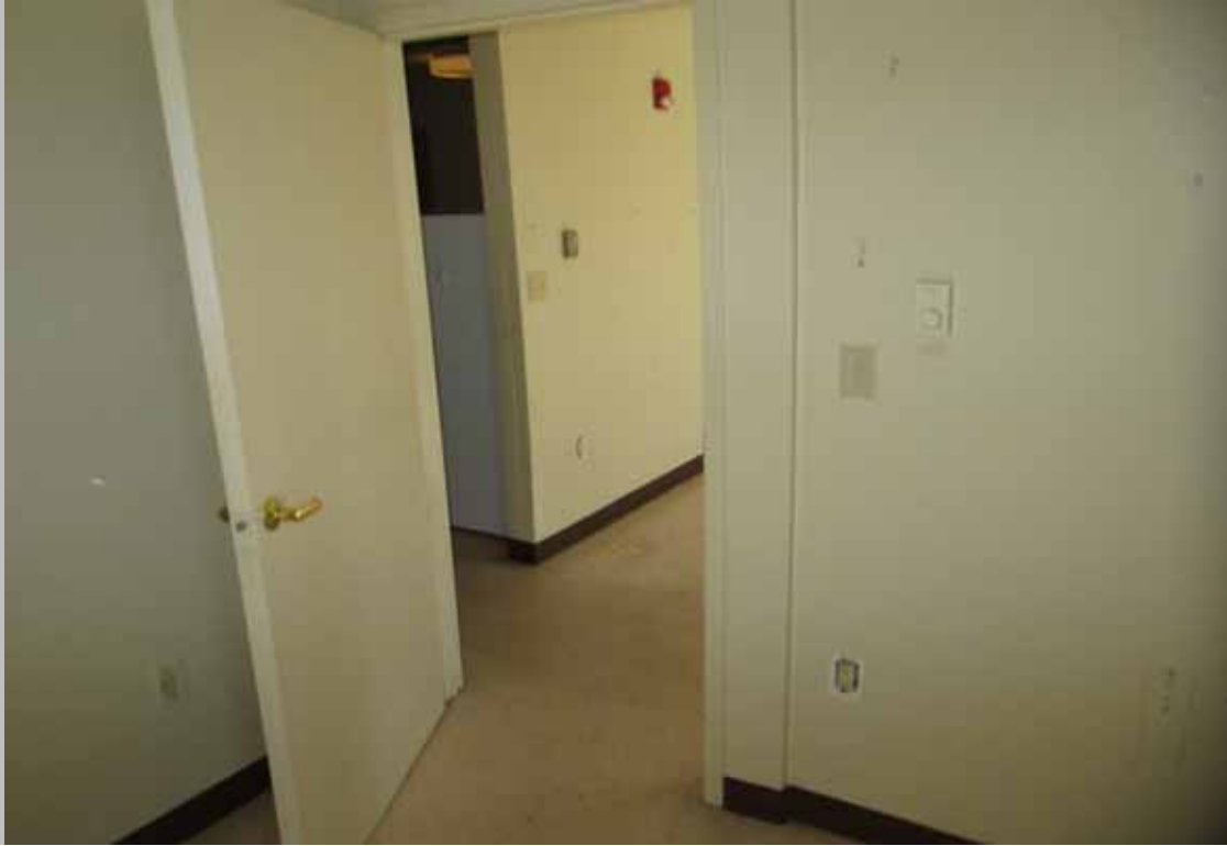
Handicapped unit bedroom door with levered hardware
