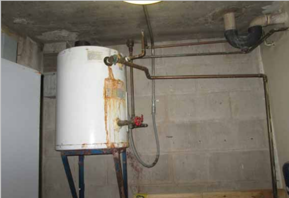
Mechanical electric hot water heater beyond EUL (Non-Critical Repair)
