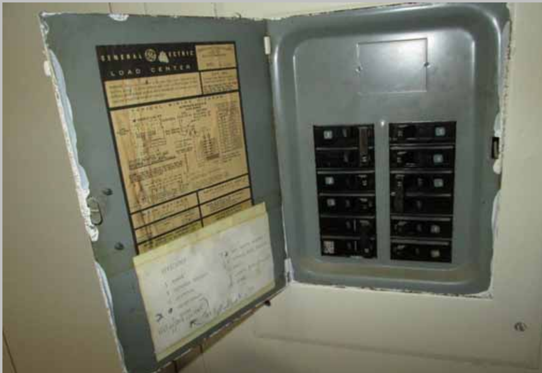
Typical GE electrical breaker panel
