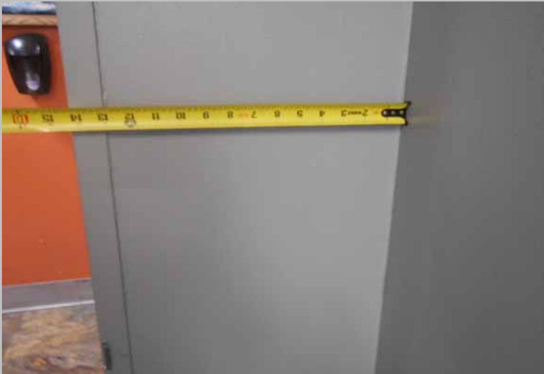
The common laundry room door does not feature 18 inches at the pull-side of the door (Critical Repair)
