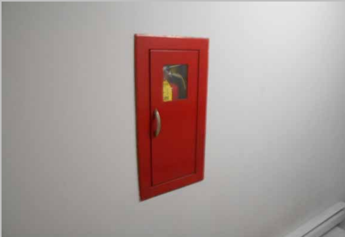
View of a fire extinguisher
