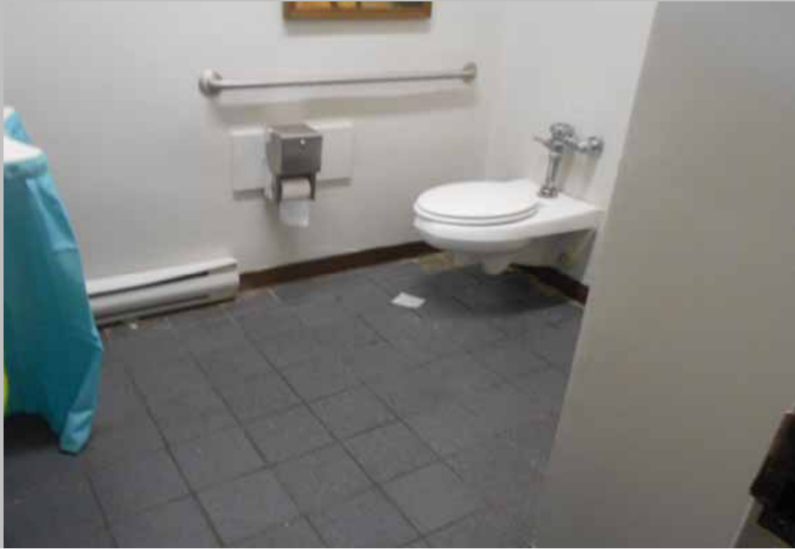
View of the men's public restroom toilet lacking a rear grab bar (Critical Repair)
