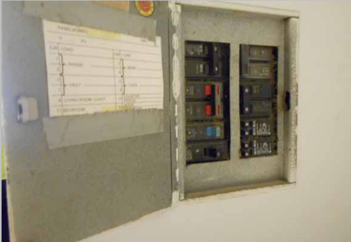
View of a Zinsco electric breaker panel - dwelling unit
