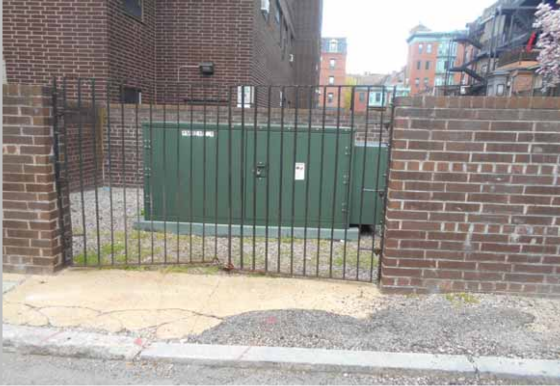
View of pad mounted electrical transformer
