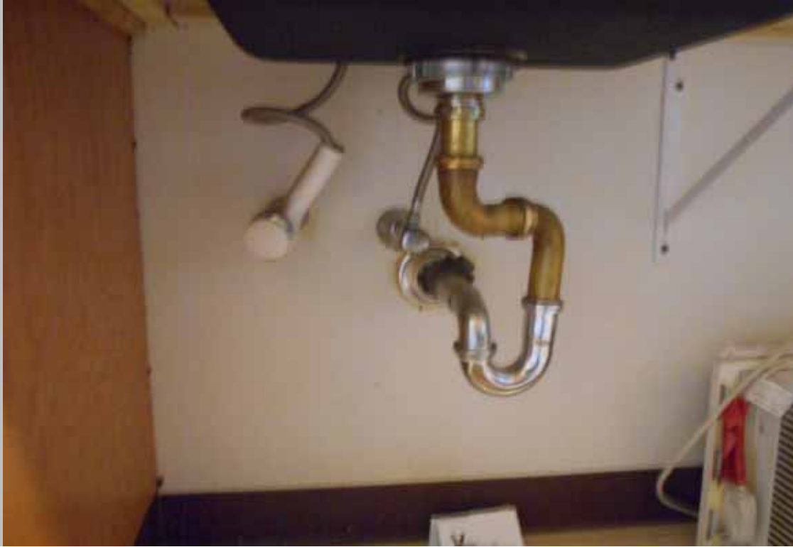
The designated handicapped dwelling unit kitchen sinks do not feature scald and abrasion protection at under-sink plumbing (Critical Repair)
