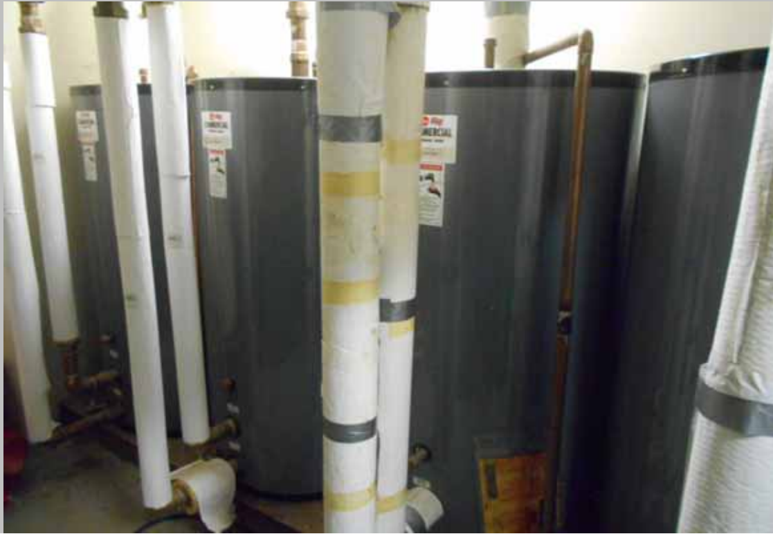
View of water storage tanks
