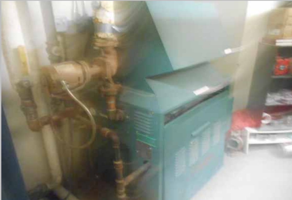
View of the DHW boiler
