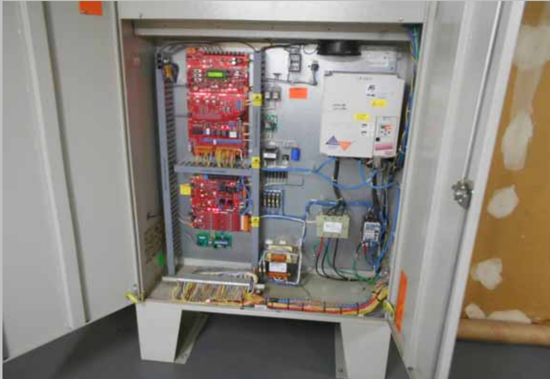
View of the elevator equipment
