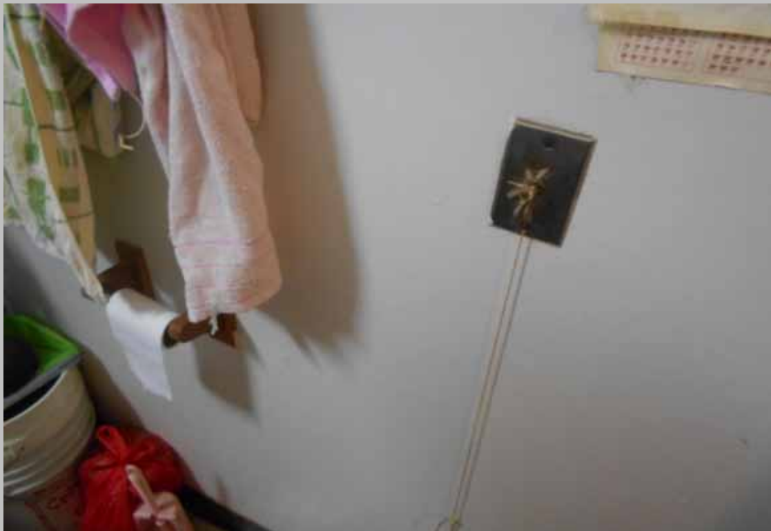
View of emergency pull cord – dwelling unit
