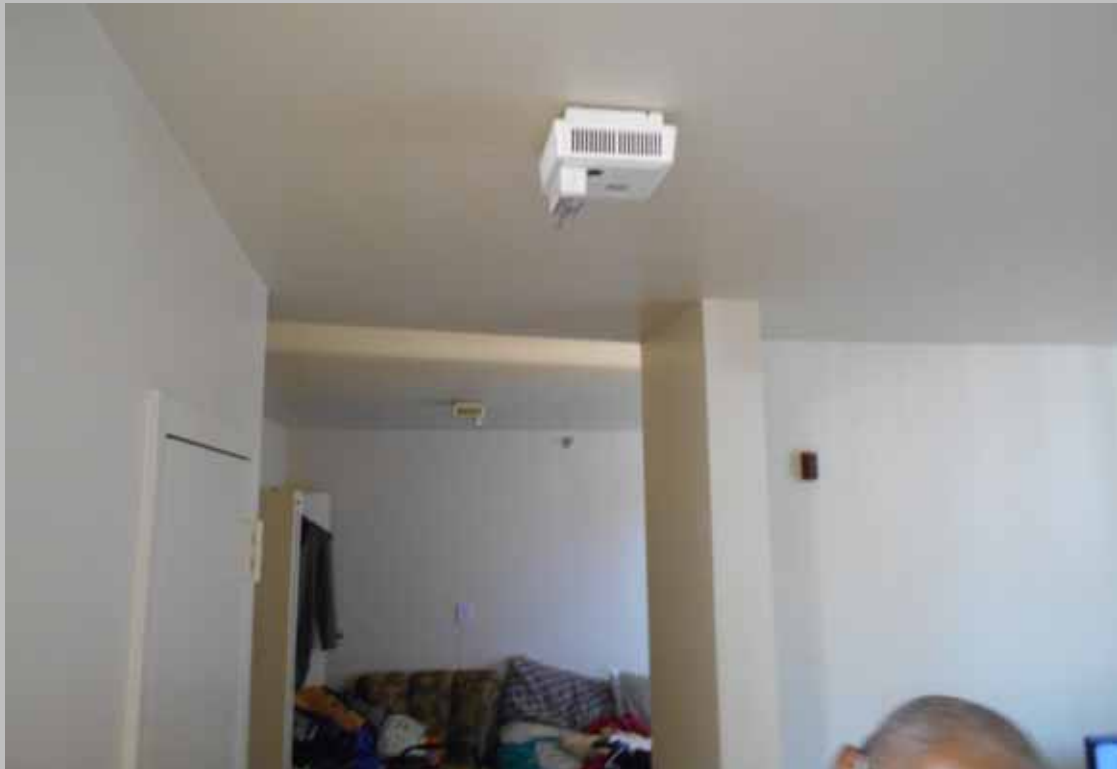
View of an A/V fire alarm – dwelling unit
