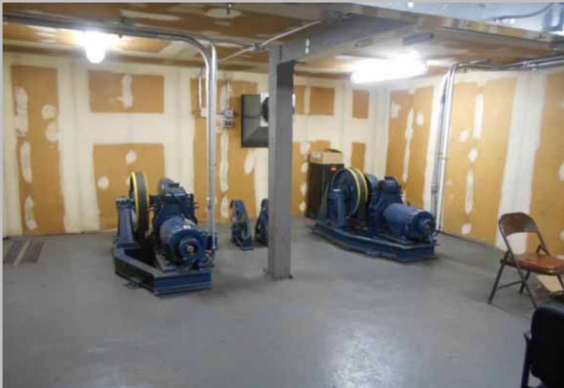
View of the elevator equipment
