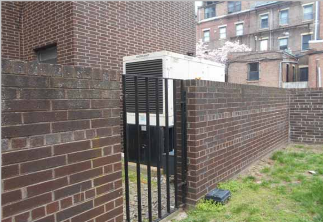
View of the generator
