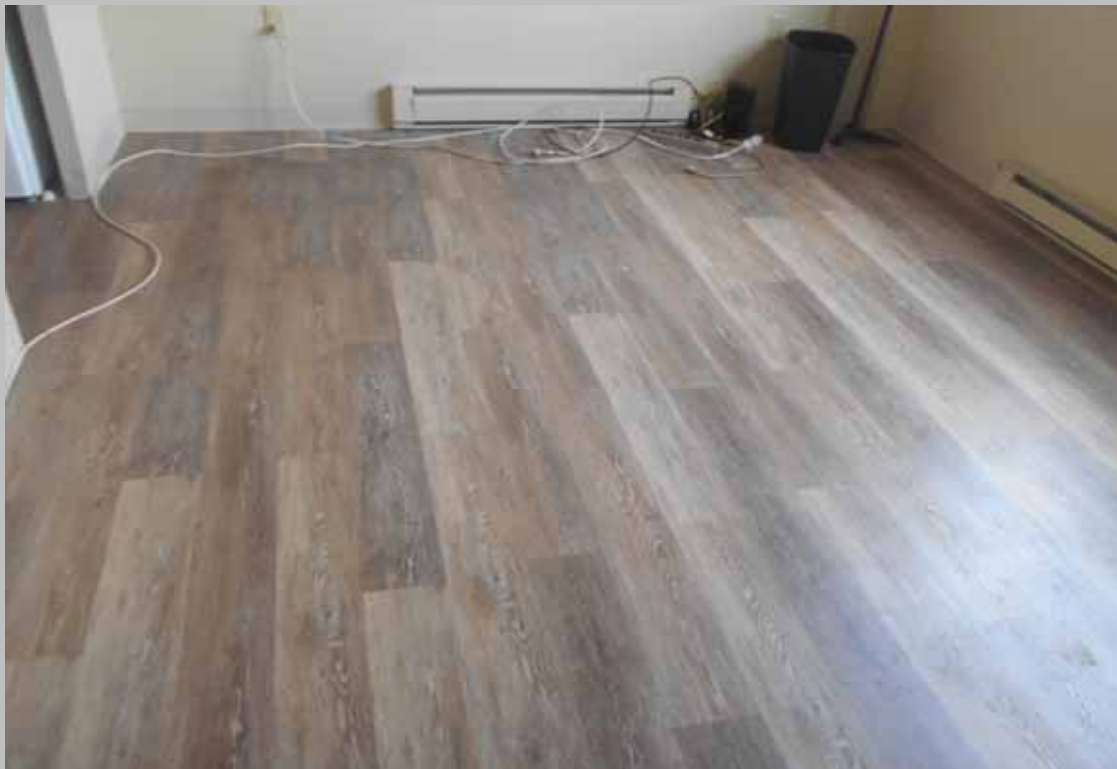
View of electric baseboard heaters - dwelling unit
