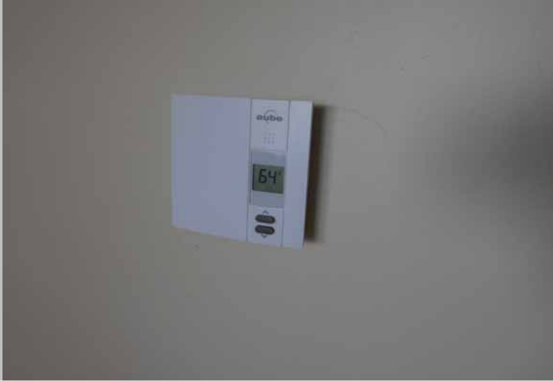
View of a thermostat – dwelling unit
