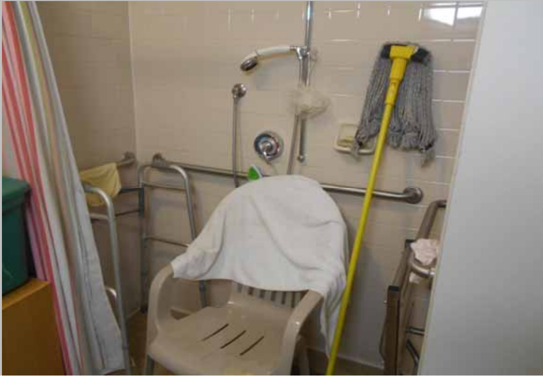
View of the bathroom within designated handicapped dwelling unit 607 – featuring a roll-in shower
