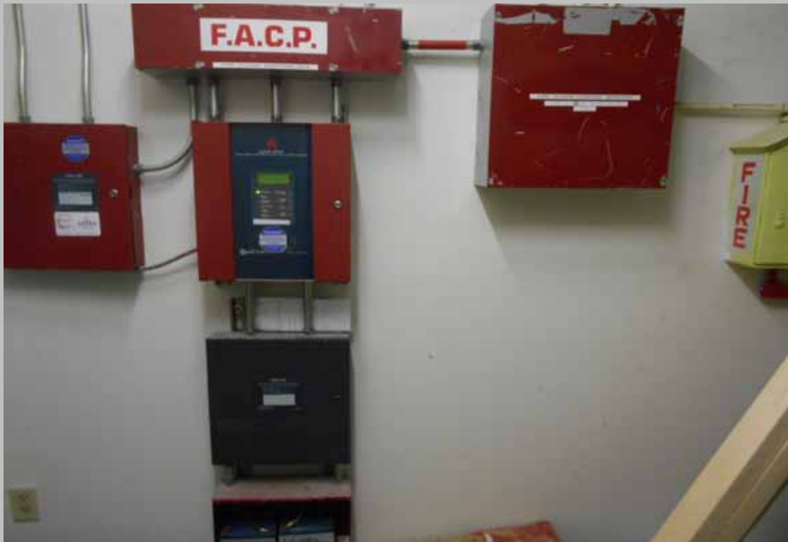
View of fire alarm control panel
