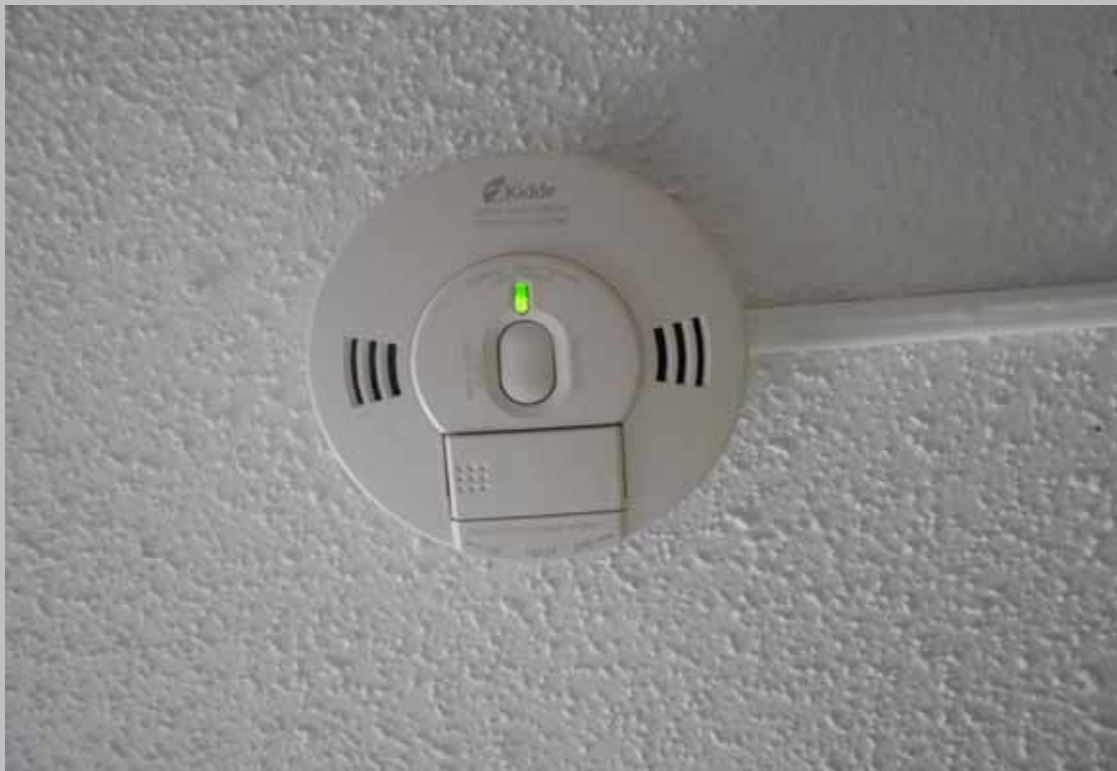
View of smoke detector - dwelling unit
