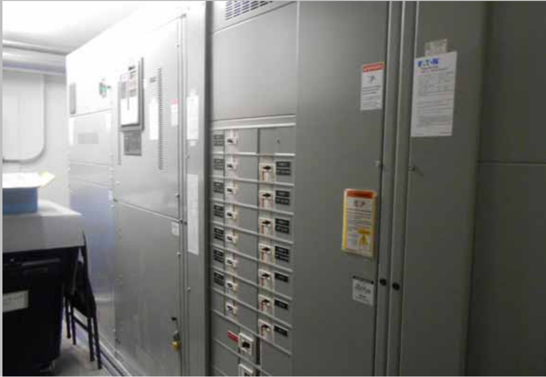
View of switchboard
