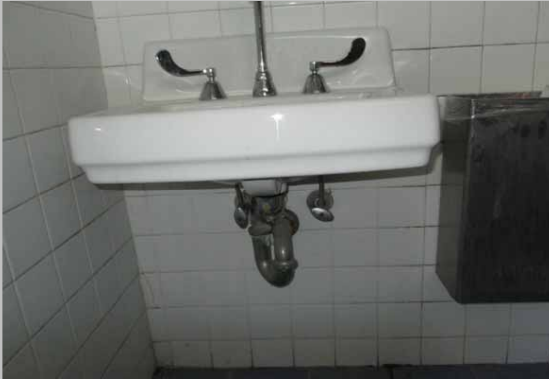
Common area restroom sink missing scald and abrasion protection on exposed piping (Critical Repairs)
