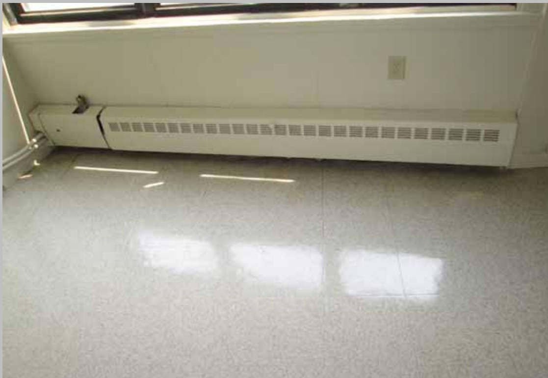
Typical dwelling unit hydronic heating
