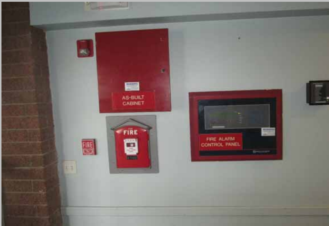
Fire alarm panels
