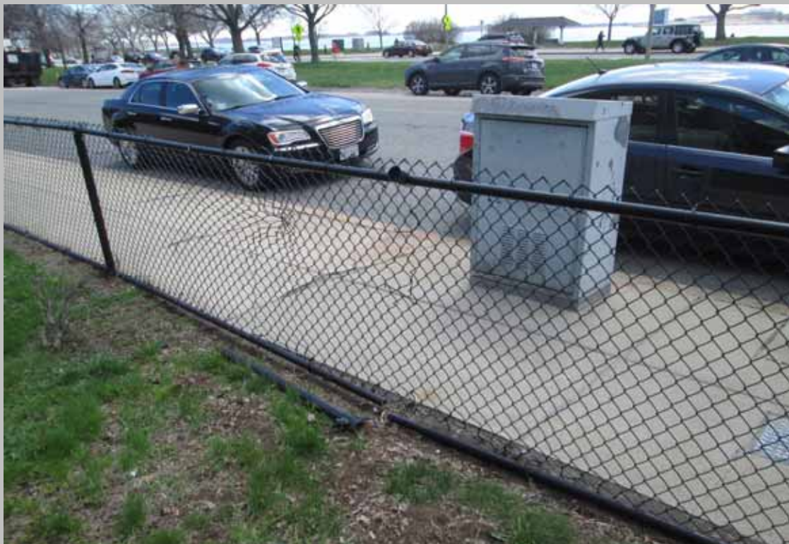
Damaged fencing (Non-Critical Repairs)
