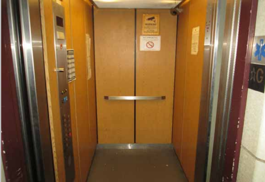
Elevator interior cab
