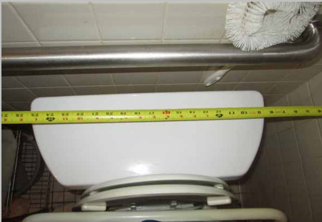
HC unit toilet centerline is not 18-inches from the adjacent wall
