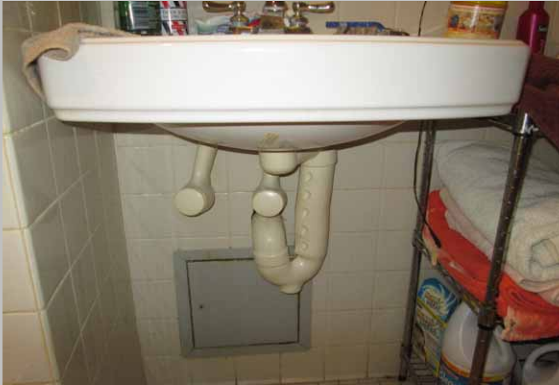
HC unit with compliant bathroom sink scald and abrasion protection
