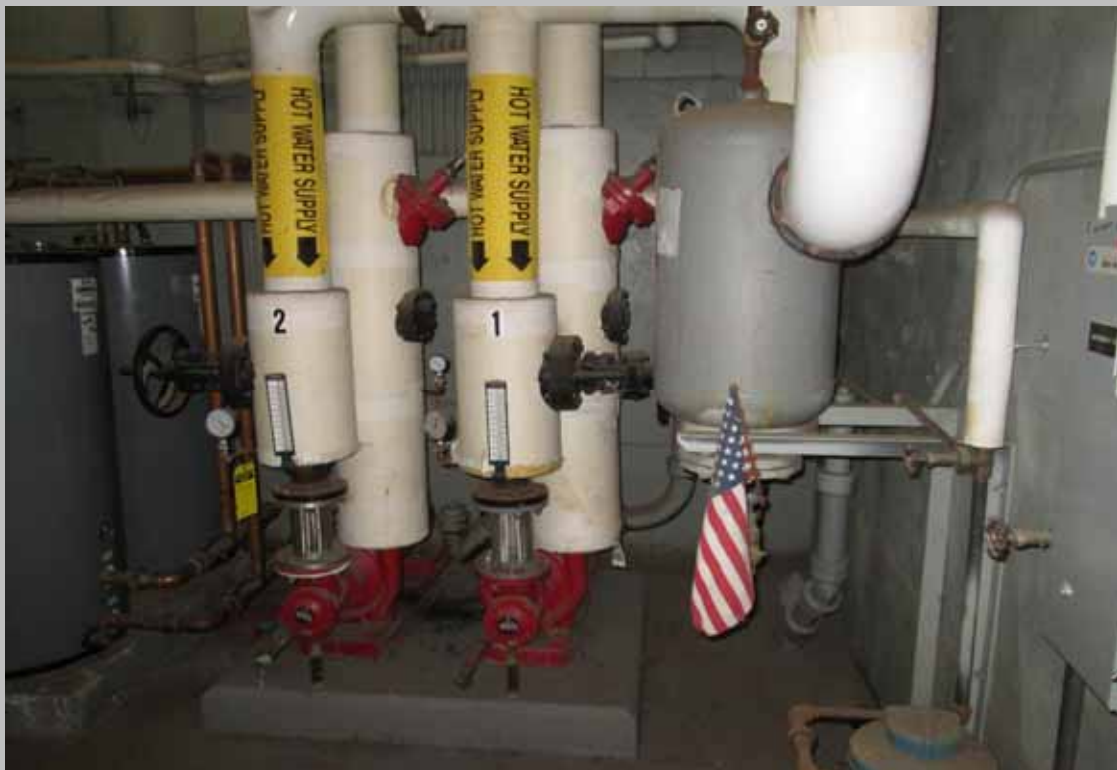
DHW circulation pumps
