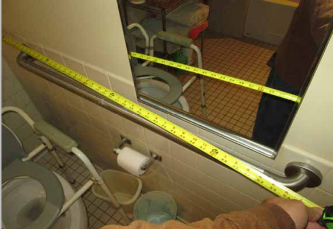
HC unit toilet with compliant side grab bar
