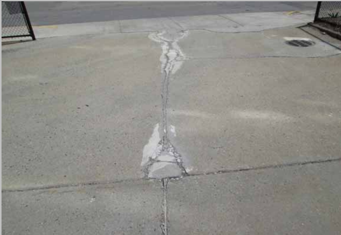
Cracked/damaged concrete (Non-Critical Repairs)
