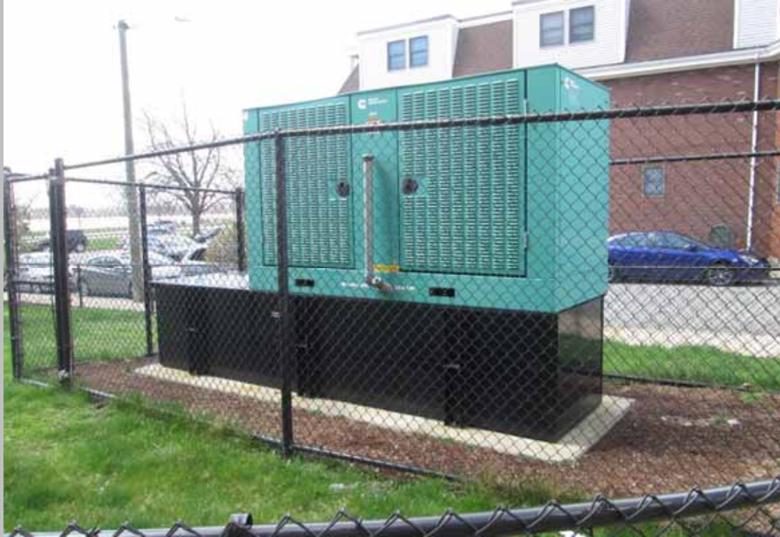
Emergency generator and AST
