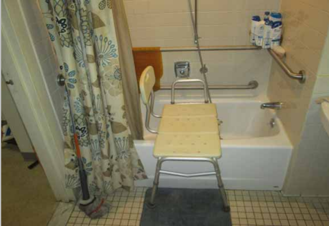
HC unit tub with compliant grab bars and levered faucet hardware
