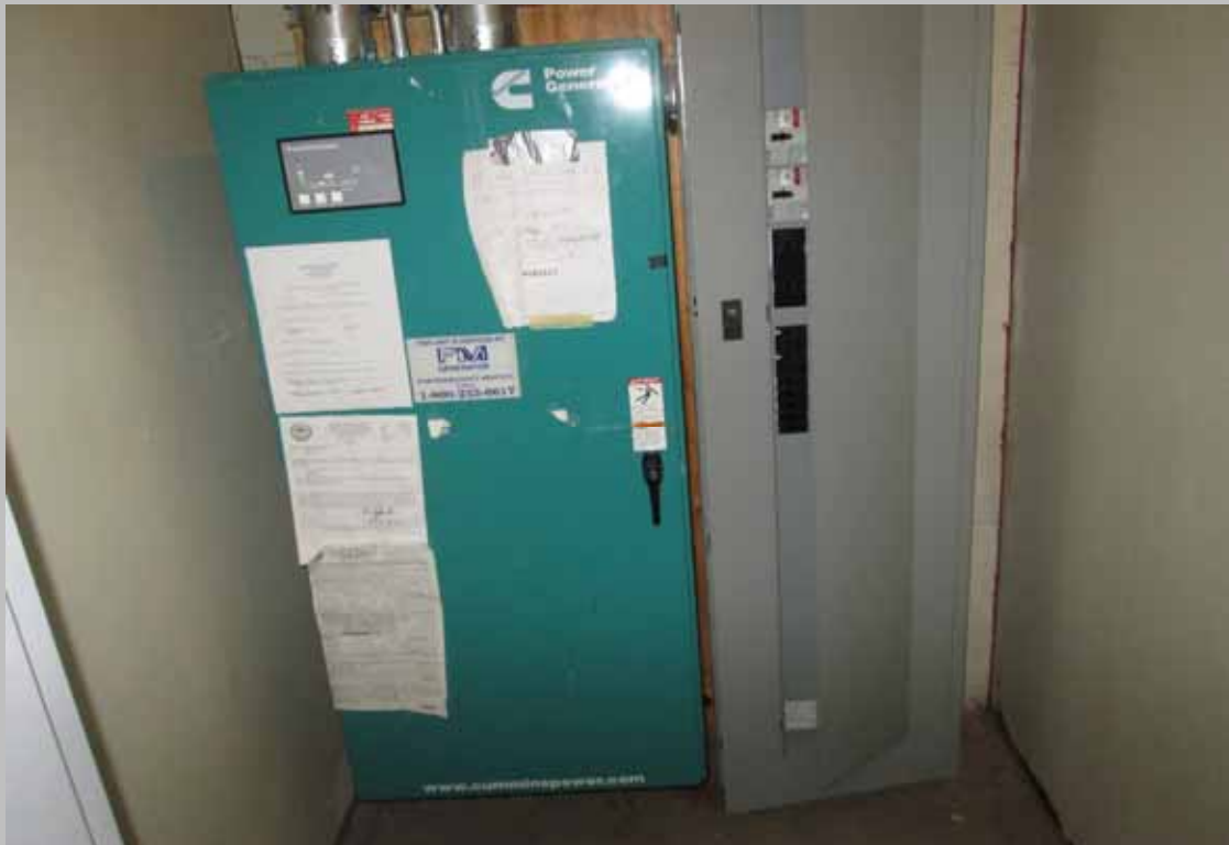
Emergency generator transfer switch
