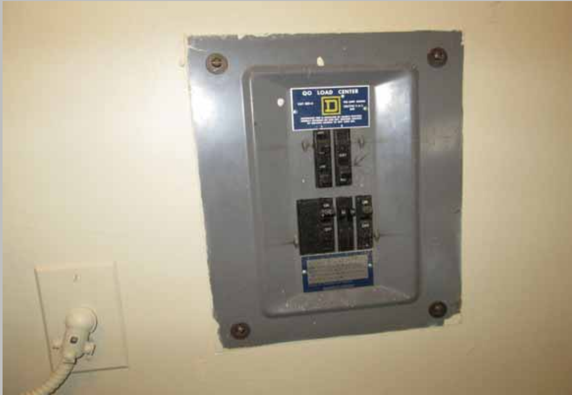
Typical dwelling unit breaker panel
