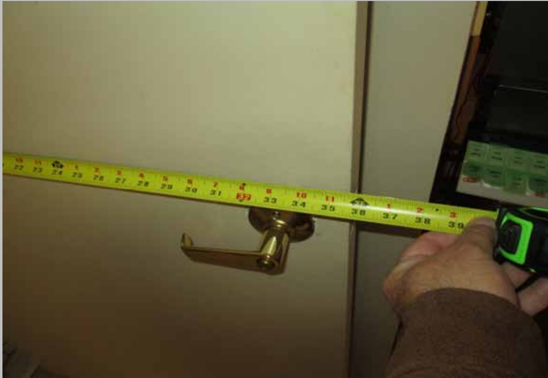
HC unit with compliant interior door
