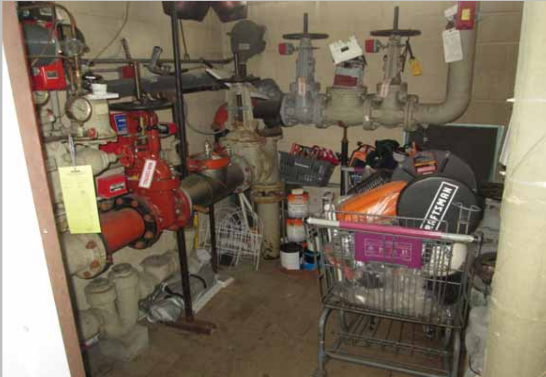
Fire pump room
