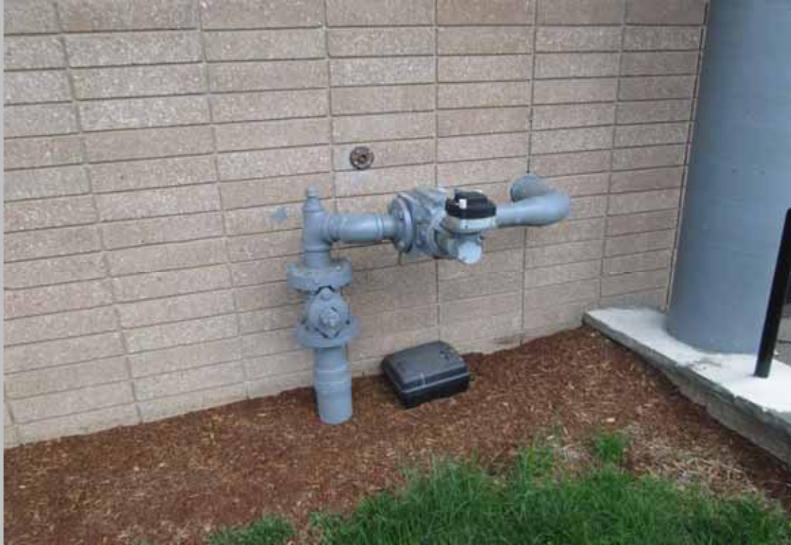
Natural gas meter
