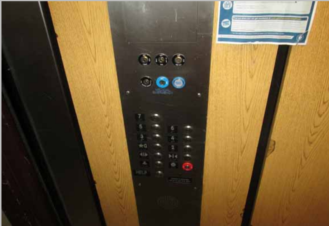
Elevator cab controls with ADA and fireman's controls
