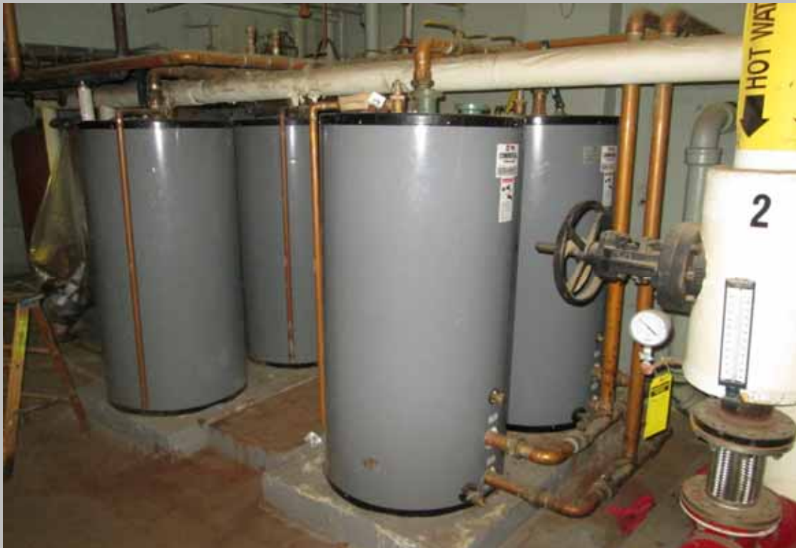
Rheem DHW commercial storage tanks
