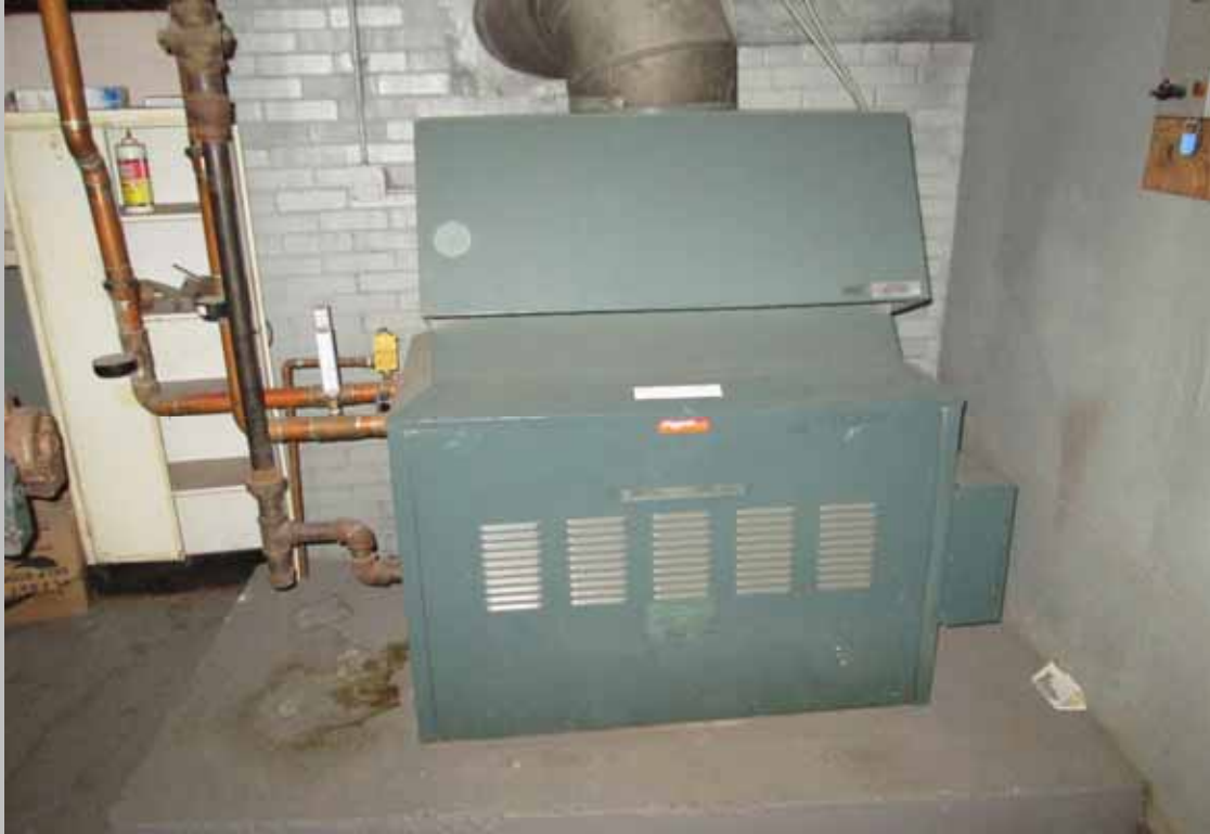
Raypack DHW boiler
