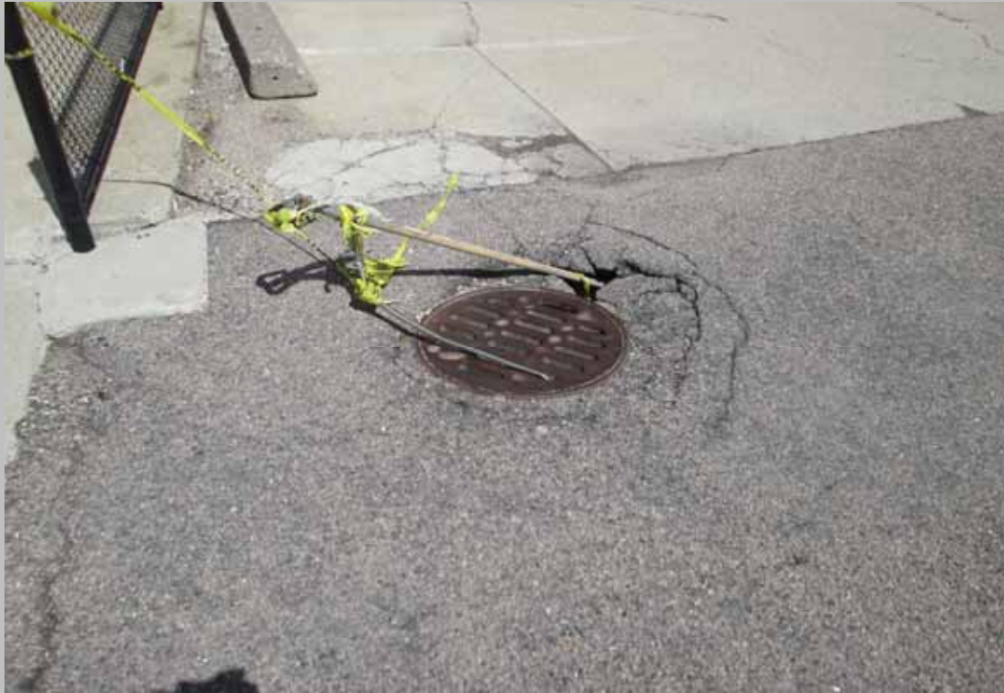
Damaged asphalt surface (Non-Critical Repairs)
