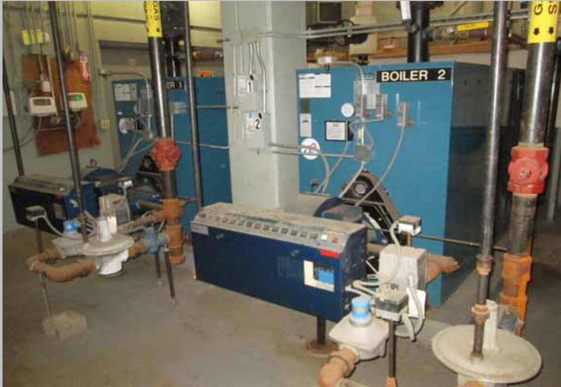
Burnham heating boilers
