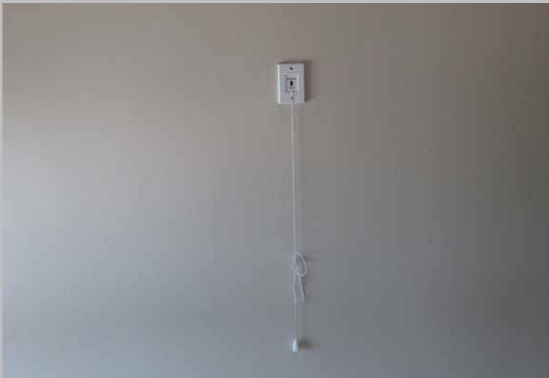
View of emergency pull cord - dwelling unit
