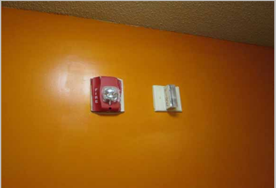
View of fire alarms - dwelling unit
