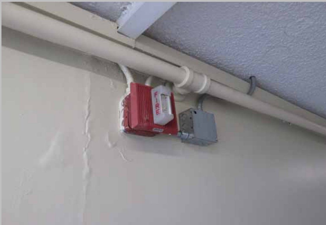
View of fire alarm
