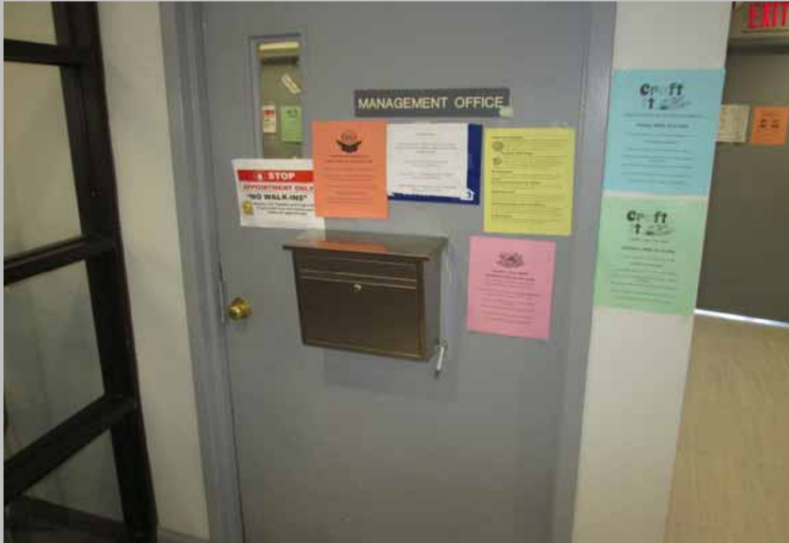
View of the public management office (leasing office) entry door lacking levered hardware (Critical Repair)
