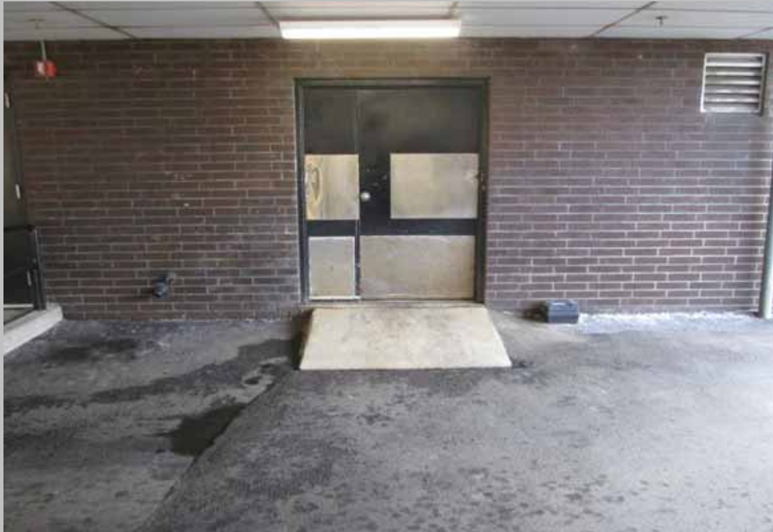
View of deteriorating brick mortar – select locations (Non-Critical Repair)
