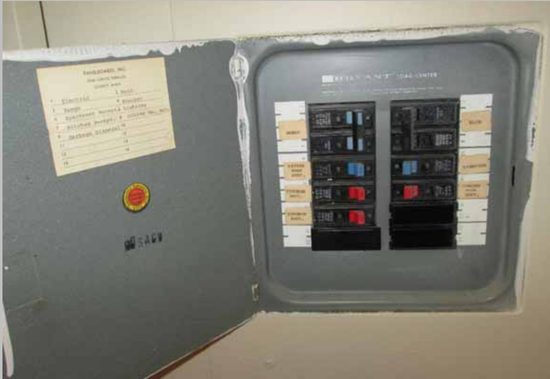
View of electric breaker panel - dwelling unit
