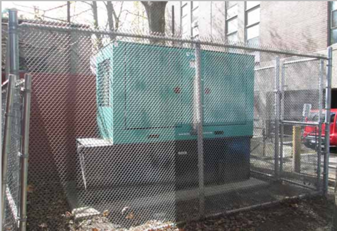
View of emergency generator
