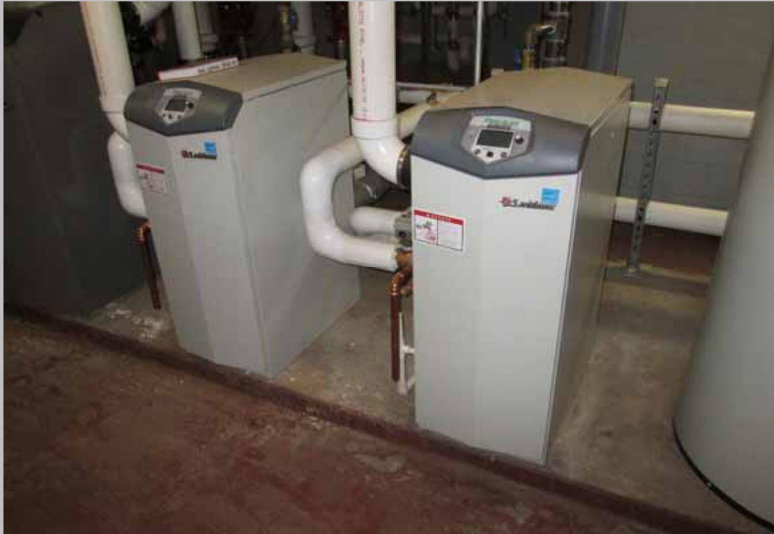
View of DHW boilers
