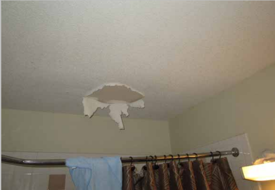
View of peeling paint in Unit 509 (Non-Critical Repair)
