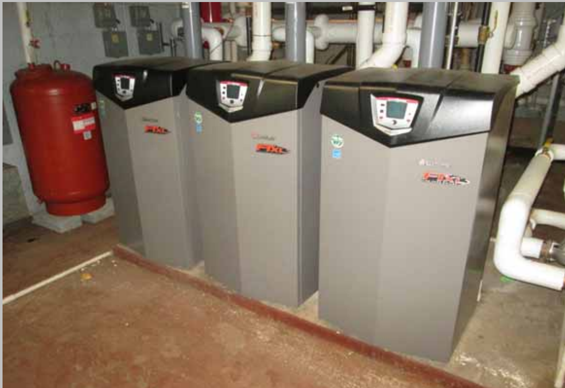
View of heating boilers
