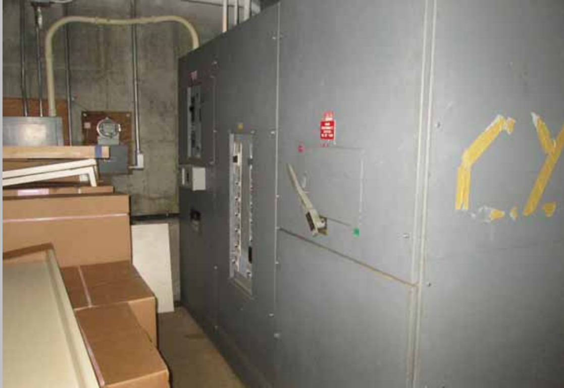
View of switchboard
