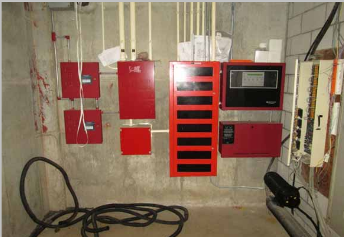
View of fire alarm control panel
