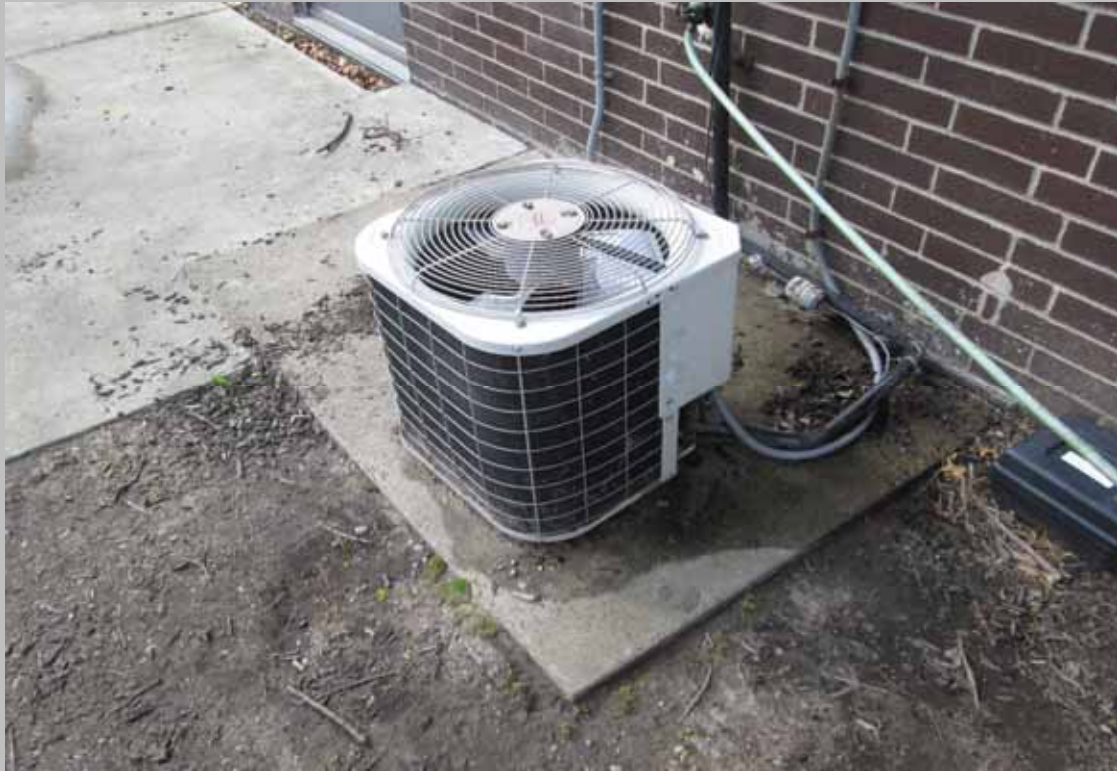
View of pad mounted condensing unit
