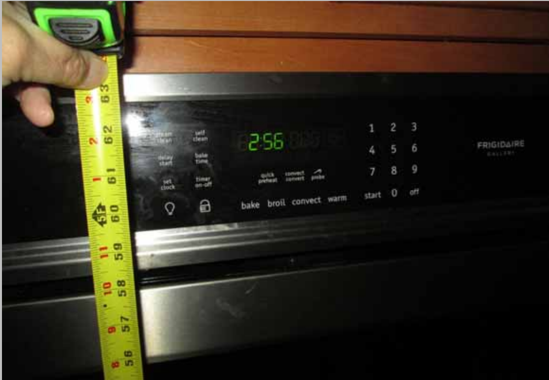
View of non-compliant height cabinet-mounted oven controls with a typical designated handicapped dwelling unit
