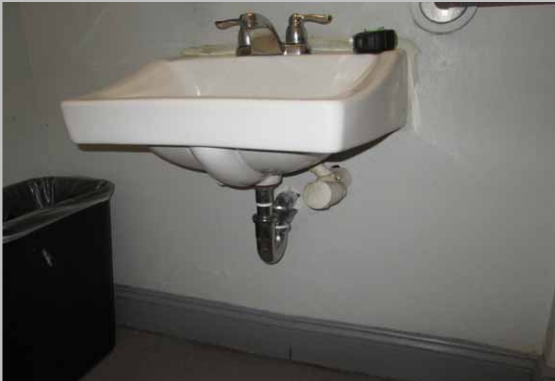
View of the common area restroom sink lacking scald and abrasion protection on piping (Critical Repair)
