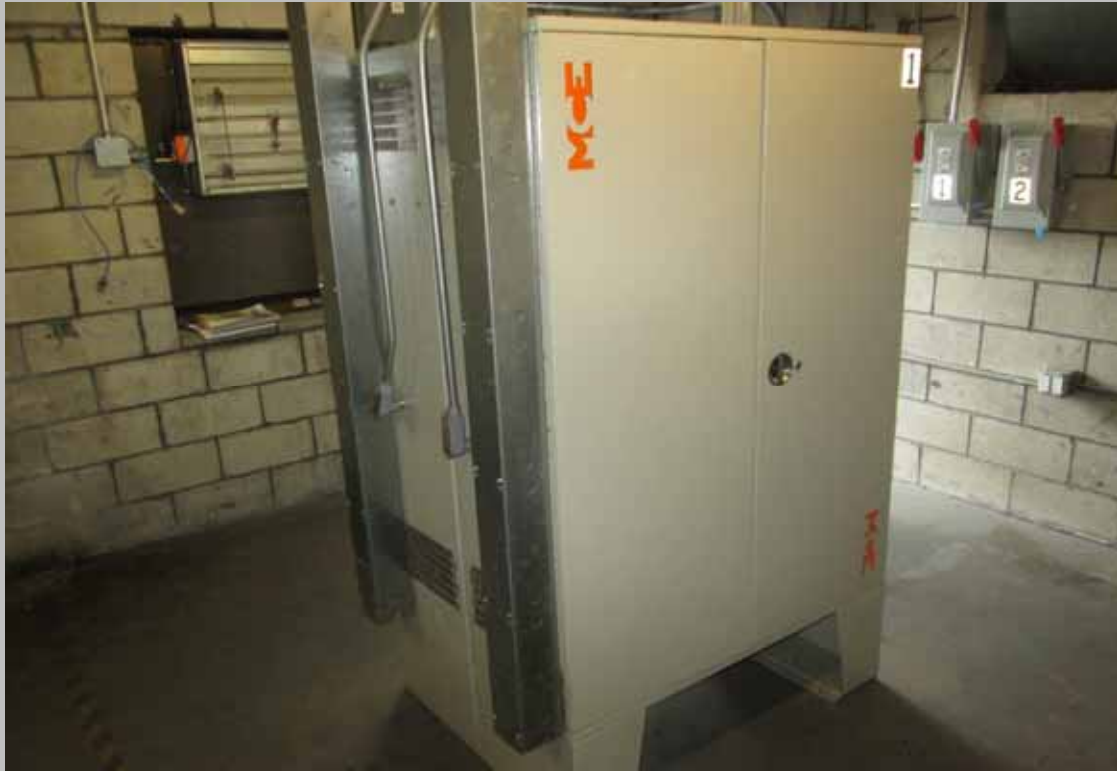
View of elevator equipment
