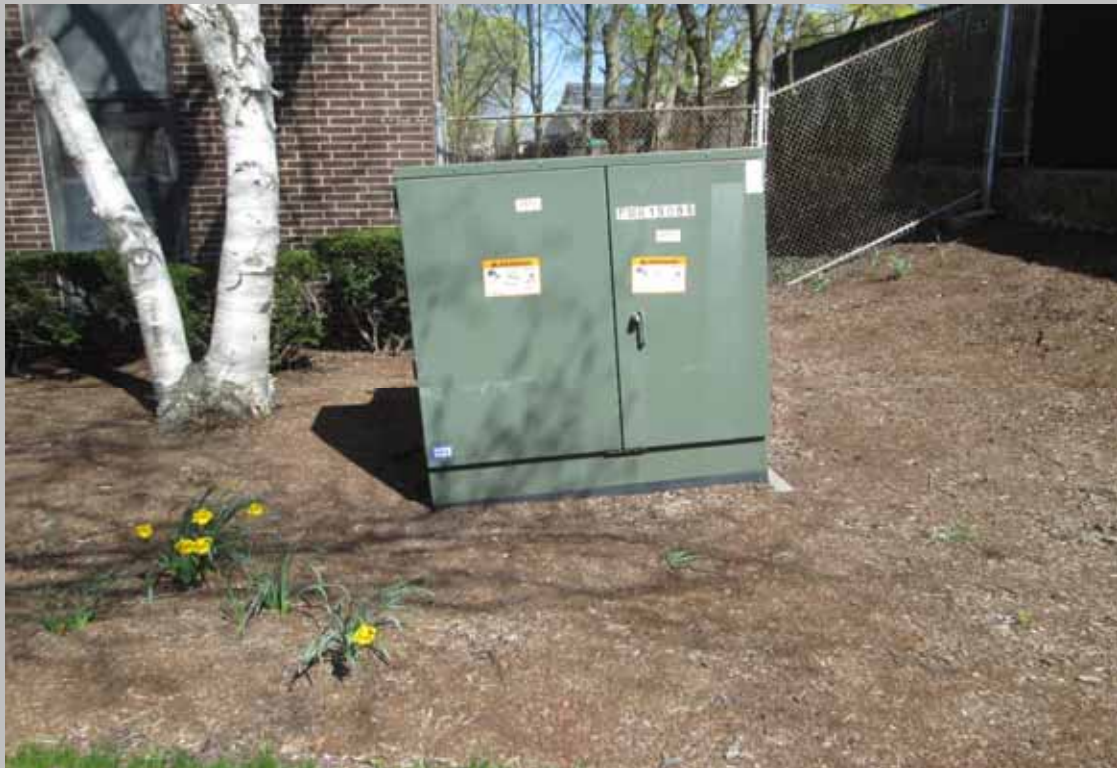
View of pad mounted electrical transformer
