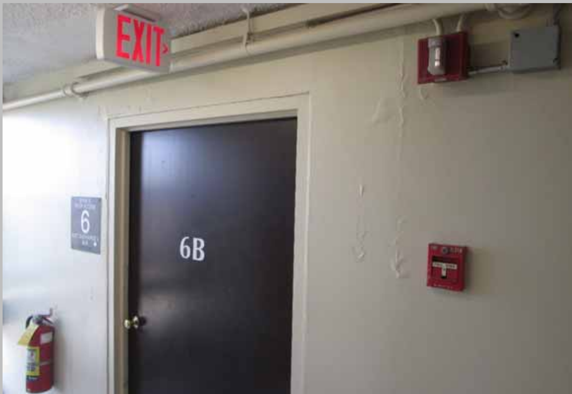
View of 6 th floor hallway damage caused from the roof leak (Non-Critical Repairs)
