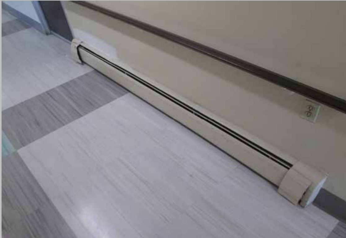
View of a common area hydronic baseboard heater
