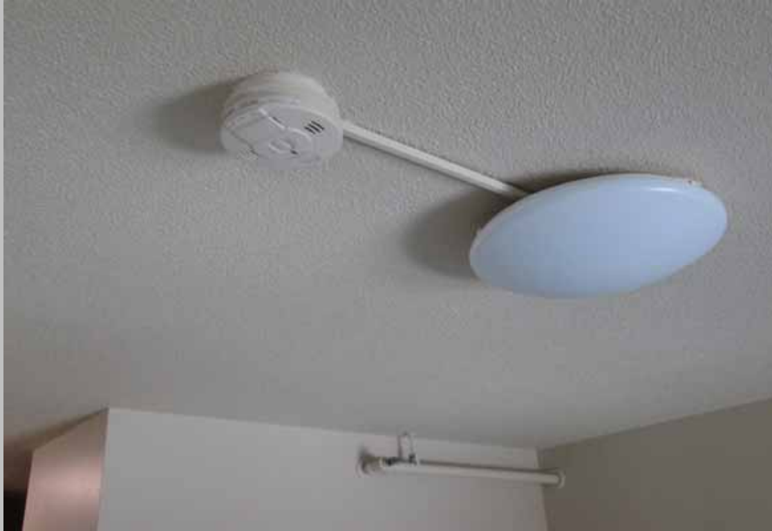
View of smoke detector - dwelling unit
