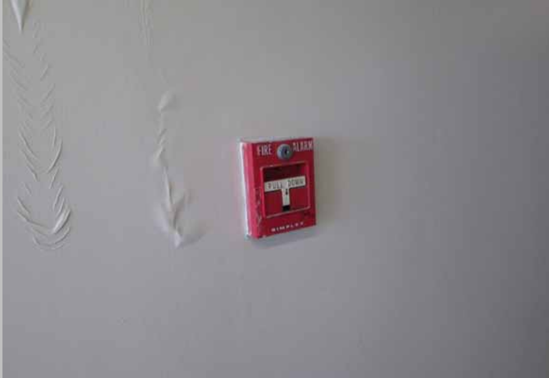
View of fire alarm pull station
