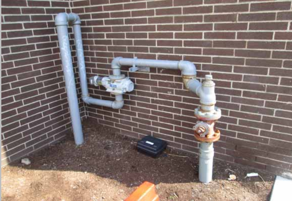
View of property metering
