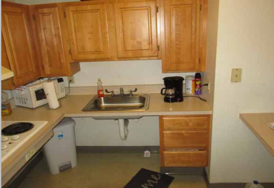
View of the kitchen within designated handicapped unit 404 featuring a roll-under sink with levered handle hardware and scald and abrasion protection and lowered upper cabinetry
