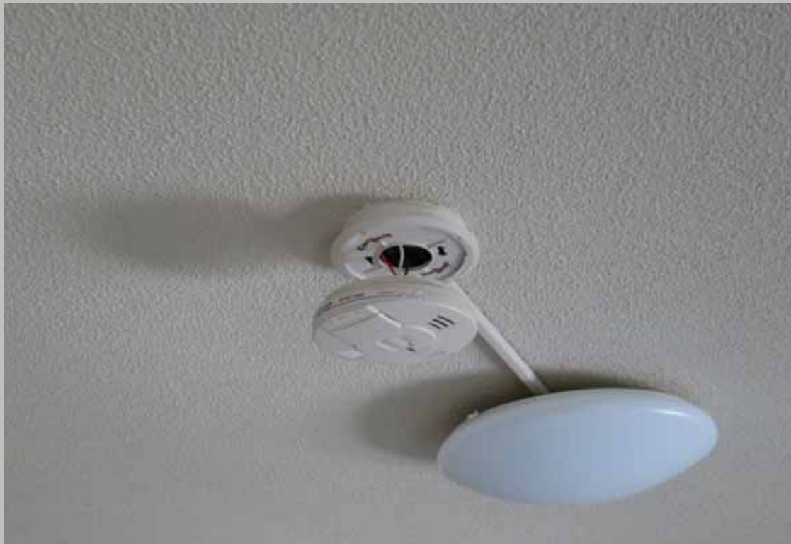
View of smoke detector - dwelling unit
