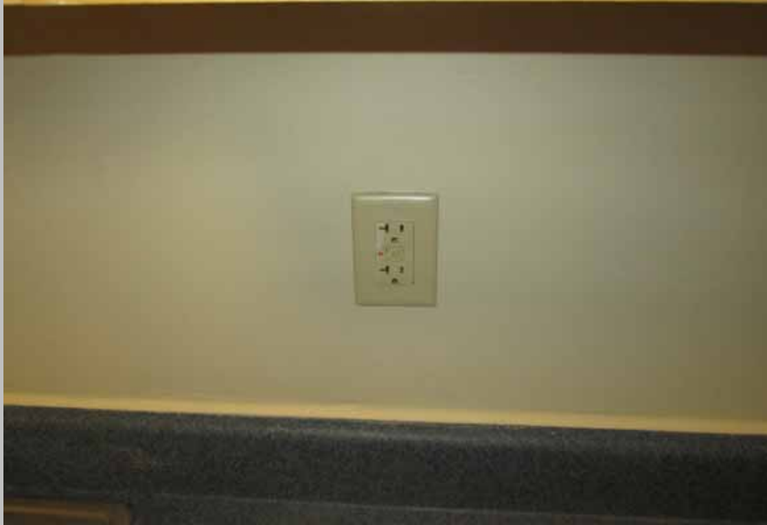
View of GFCI electrical outlet – dwelling unit
