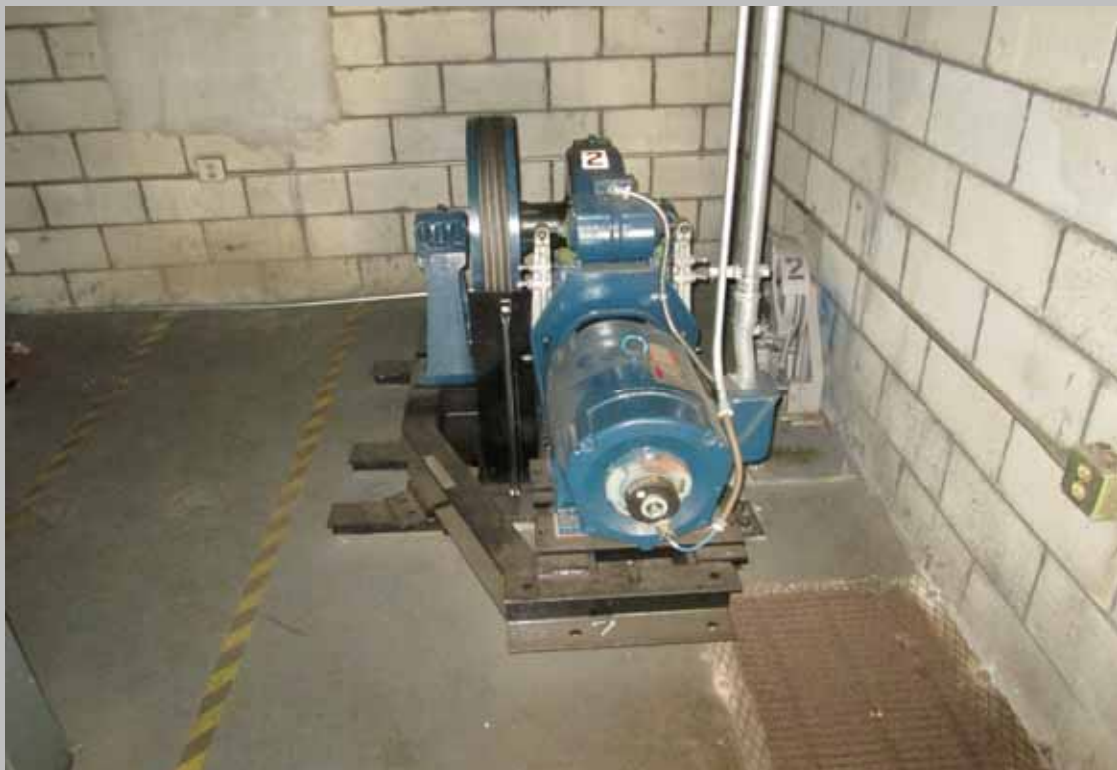
View of elevator equipment
