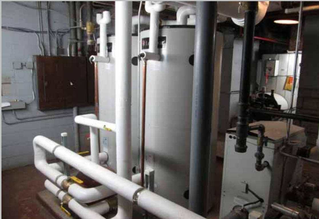
View of water storage tanks
