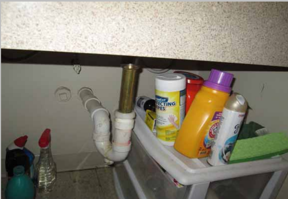
View of the kitchen sink in HC Unit 514 lacking scald and abrasion protection on piping (Critical Repairs)
