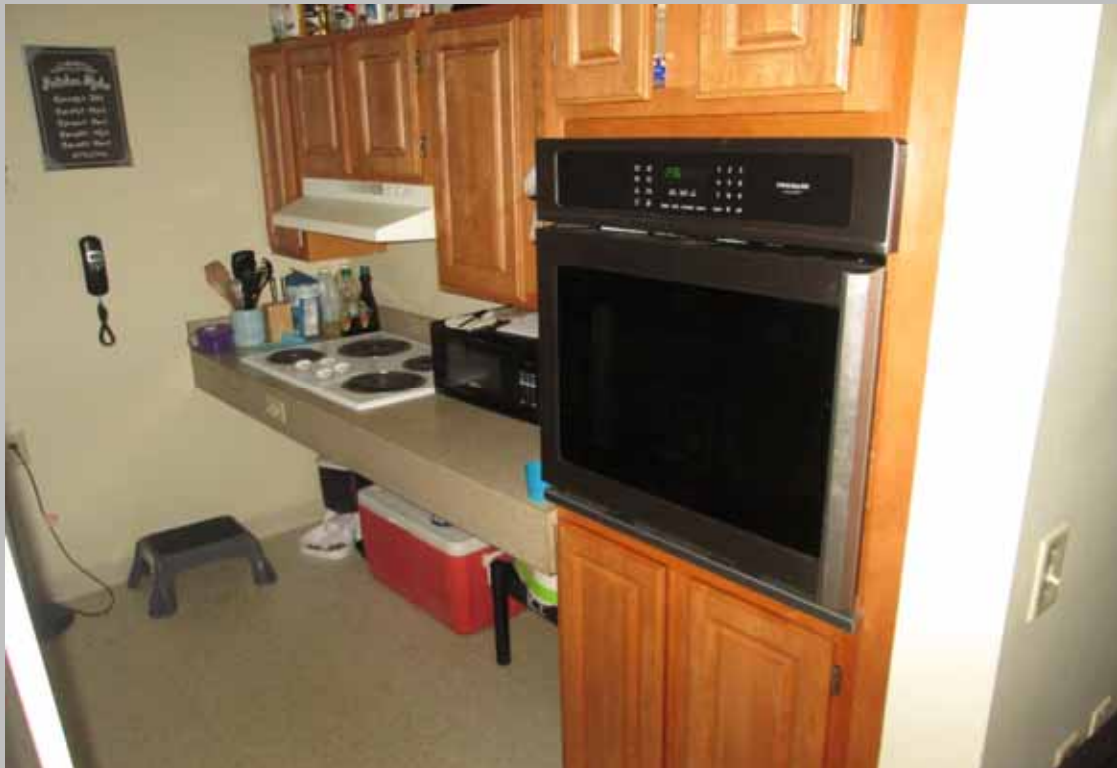
View of the kitchen within designated handicapped unit 514 featuring a roll-under cook-top
