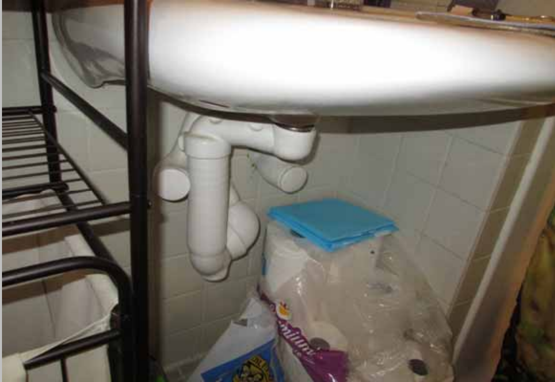
View of the bathroom sink within designated handicapped dwelling unit 514 featuring compliant scald and abrasion protection
