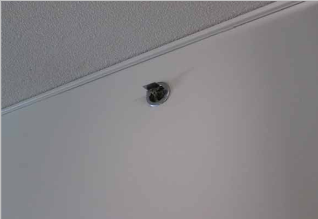
View of fire sprinkler head – dwelling unit
