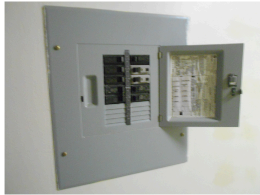
Building 1 unit 238, 1br/1ba - Tenant electrical breaker
