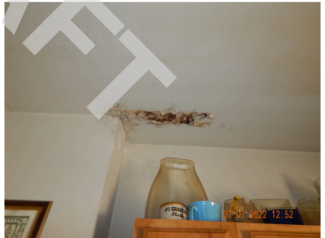
124. Mold, leak in Unit 1013
