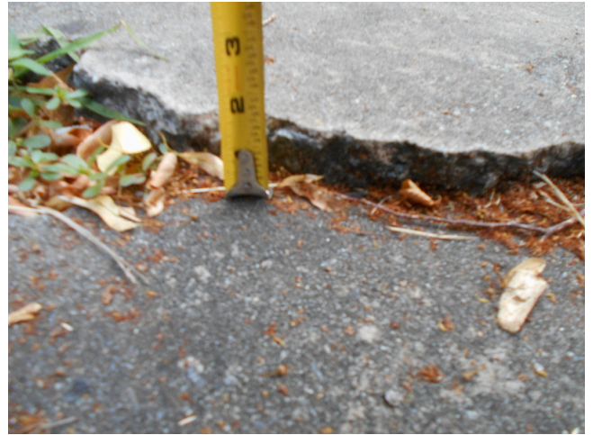
126. Concrete trip hazard by building 3 (Critical Repair)
