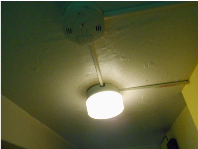
55. Building 2 unit 222, 2br/1ba - Living area smoke detector
