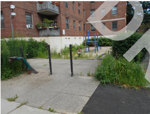
Playground by building 22, overgrown (Non-Critical Repair)
