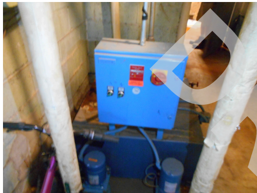
Leasing office boiler pump
