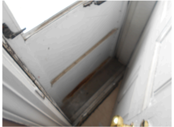
118. Building 5 unit 186, 64 O'Callaghan Way, 3br/1ba Townhouse - Rear door, damaged (Non-Critical Repair)
