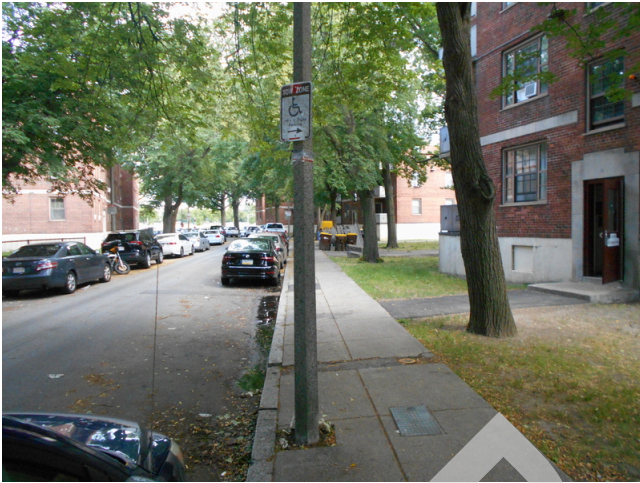
45. Building 3 handicap street parking, no curb cut or access aisle (Critical Repair)
