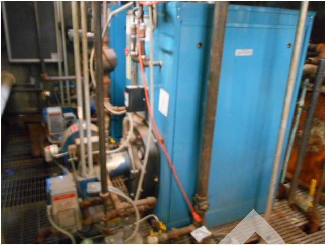
65. Building 4 mechanical room boilers
