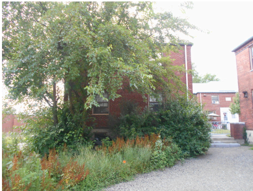
Building 5 side façade, foliage growing along building façade (Non-Critical Repair)
