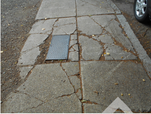
81. Concrete sidewalk by building 7, damaged (Critical Repair)
