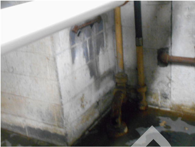
61. Building 1 basement water intrusion (Critical Repair)
