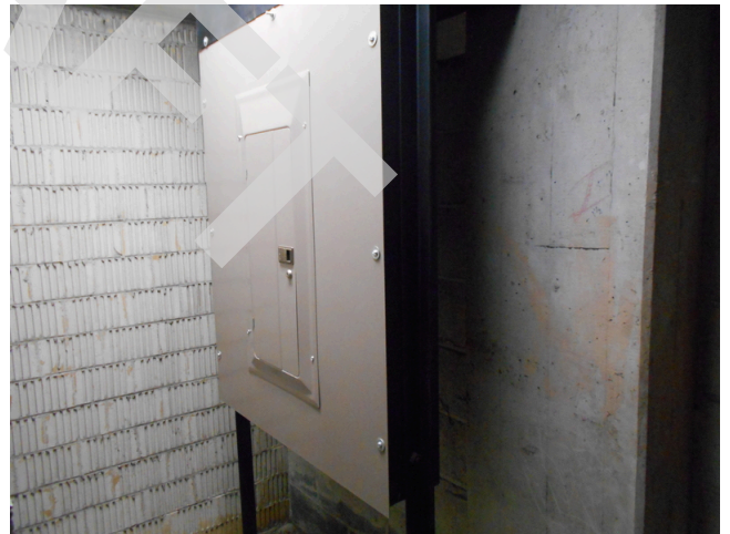
56. Building 1 basement electrical panel
