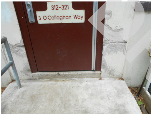
3 O'Callaghan way entrance, damaged entry (Non-Critical Repair)
