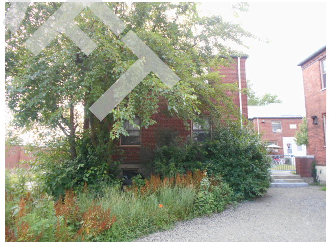
108. Building 5 side façade, foliage growing along building façade (Non-Critical Repair)
