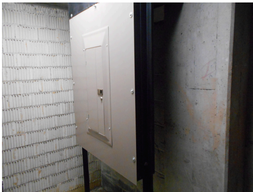
Building 1 basement electrical panel
