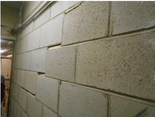
167. Building 30 basement, 15 Logan way, cracking CMU-wall (Non-Critical Repair)
