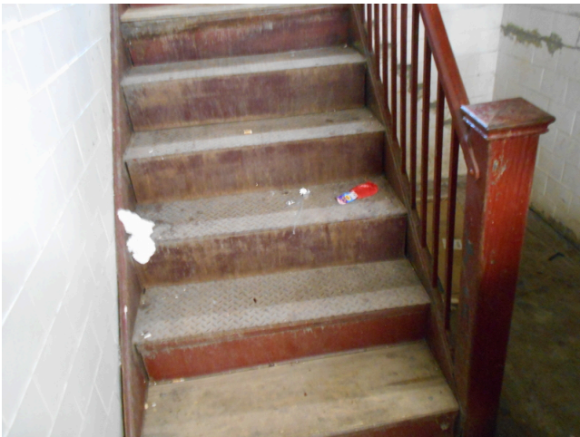
155. Building 32, 37 Logan way stairwell, damaged stairs (Non-Critical Repair)
