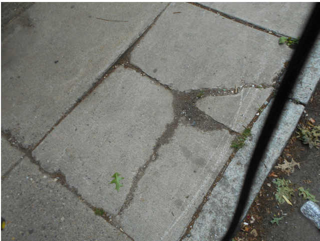
115. Concrete trip hazard between building 3 and building 4 (Critical Repair)
