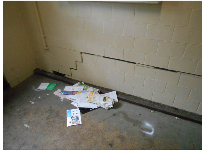
178. Building 17 basement, cracked (Non-Critical Repair)
