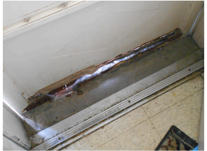
86. Building 4 unit 201, 34 O'Callaghan Way, 2br/1ba Townhouse - rear door (Non-Critical Repair)
