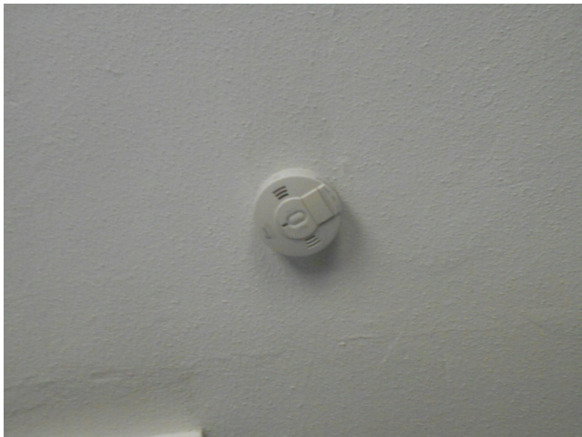
275. Community building, task force headquarters, smoke detector
