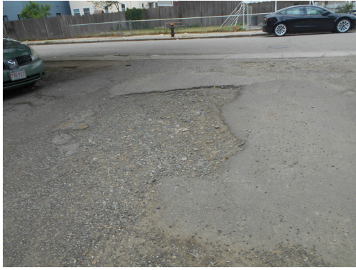
Asphalt parking lot by building 30, damaged (Non-Critical Repair)
