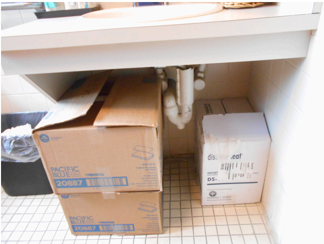
23. Leasing office public restroom sink scald abrasion protection
