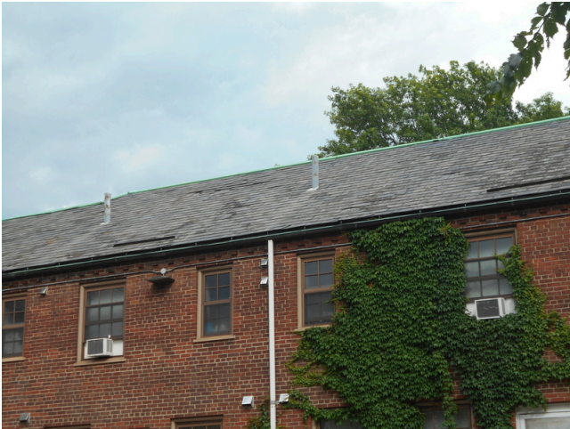
99. Building 6 slate tile roofing, shingles falling (Non-Critical Repair)
