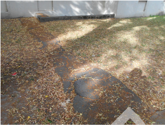
141. Building 12 side façade asphalt walkway, cracked (Non-Critical Repair)
