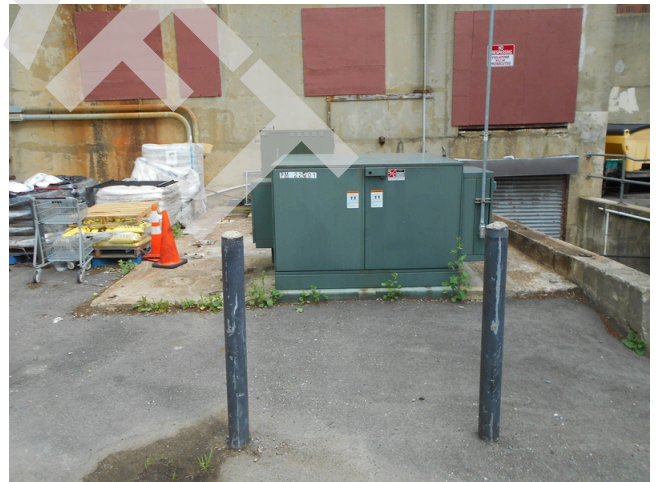
80. Pad mounted electrical transformers
