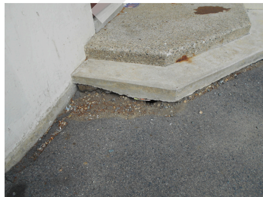
Building 32, 33 Logan way stairwell entrance, Concrete stairs at entrance eroded (Non-Critical Repair)
