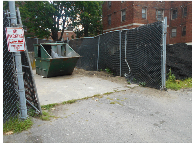
198. Refuse area by building 30, damaged fencing (Non-Critical Repair)
