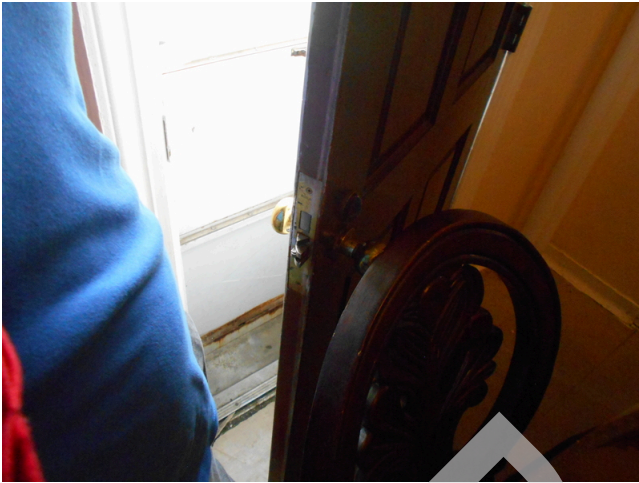
117. Building 5 unit 186, 64 O'Callaghan Way, 3br/1ba Townhouse - Rear door, damaged (Non-Critical Repair)
