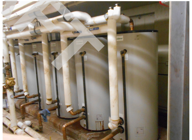
160. Building 32 boiler room hot water tanks
