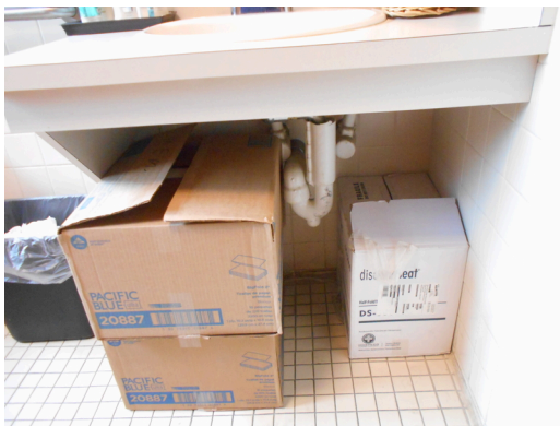
Leasing office public restroom sink scald abrasion protection
