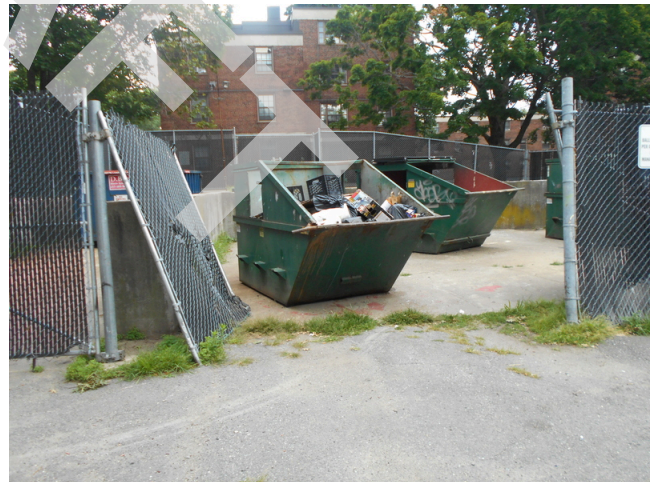
196. Refuse area by building 30, damaged fencing (Non-Critical Repair)
