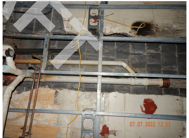
132. Units 1016 and 915 have fire damage
