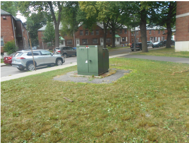
243. Pad mounted electrical transformer
