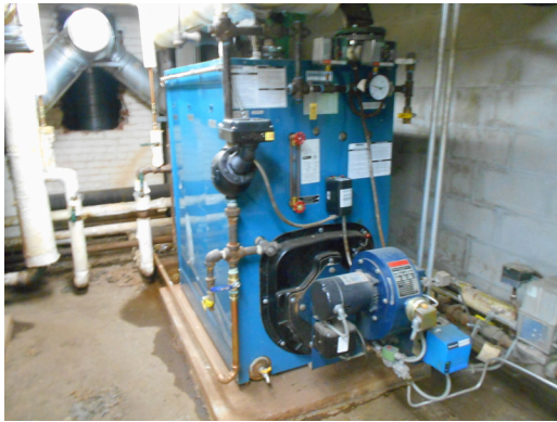
Building 32 boiler room
