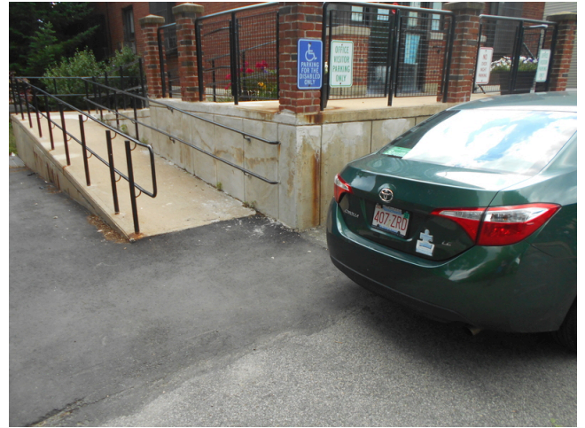
70. Leasing office accessible parking space sign, no parking space markings, no access aisle, no horizontal signage (Critical Repair)
