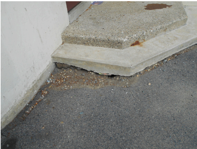
215. Building 32, 33 Logan way stairwell entrance, Concrete stairs at entrance eroded (Non-Critical Repair)
