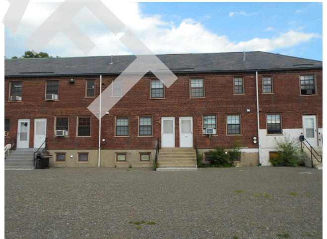
112. Building 4 rear façade, poor condition slate tile (Non-Critical Repair)
