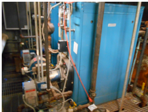
Building 4 mechanical room boilers
