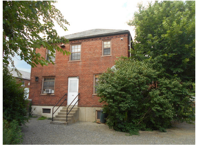
110. Building 4 side façade, foliage growing along building façade (Non-Critical Repair)
