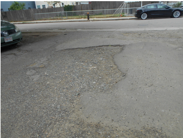
203. Asphalt parking lot by building 30, damaged (Non-Critical Repair)
