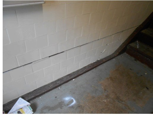
Building 17 basement, cracked (Non-Critical Repair)
