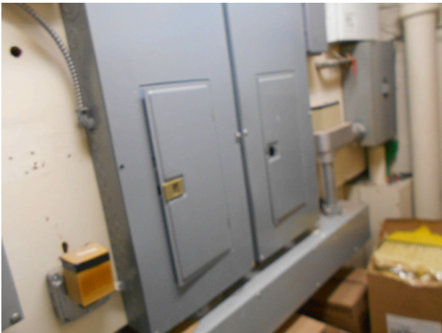
39. Leasing office electrical panel
