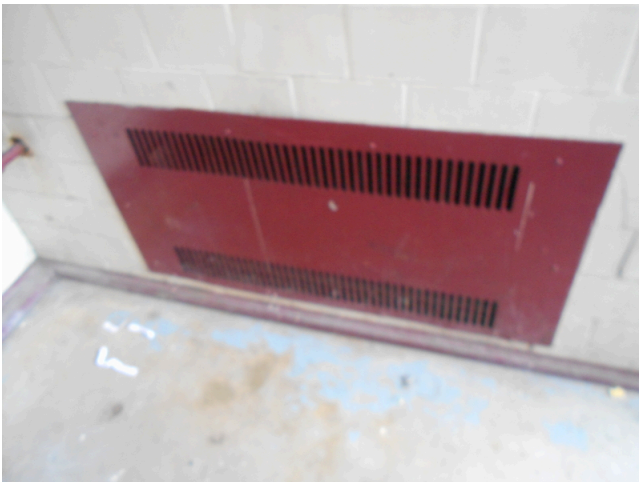
51. Typical Walk-up radiator in stairwell
