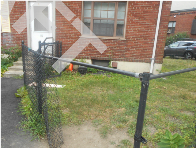
248. Damaged chain link fencing by 16 Kemp Street, unit 116 (Non-Critical Repair)
