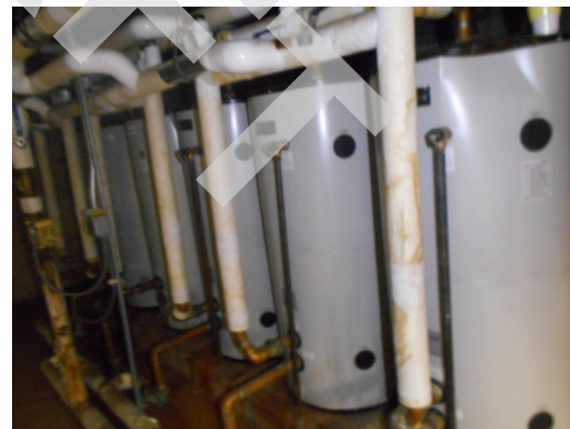
Building 30 basement, hot water tank
