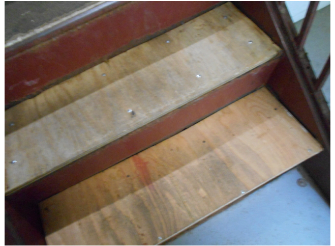
154. Building 32, 37 Logan way stairwell, damaged stairs (Non-Critical Repair)
