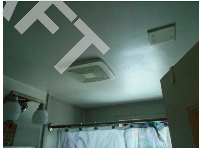
92. Building 4 unit 201, 34 O'Callaghan Way, 2br/ 1ba Townhouse - Bathroom ceiling
