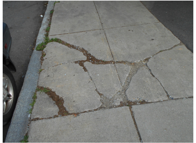
114. Concrete trip hazard between building 3 and building 4 (Critical Repair)
