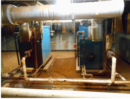
Building 17 basement boiler room, water pooling (Non-Critical Repair)
