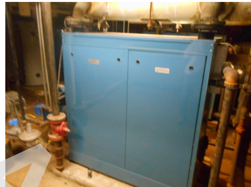
Building 30 basement, boiler
