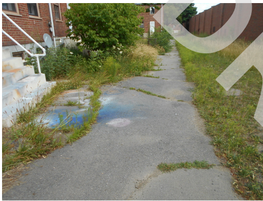
Building 3 rear façade, asphalt pathway overgrown and cracked (Non-Critical Repair)
