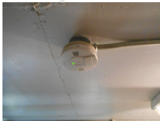
Building 3 unit 204, 28 O'Callaghan Way, 3br/1ba Townhouse - Basement smoke detector
