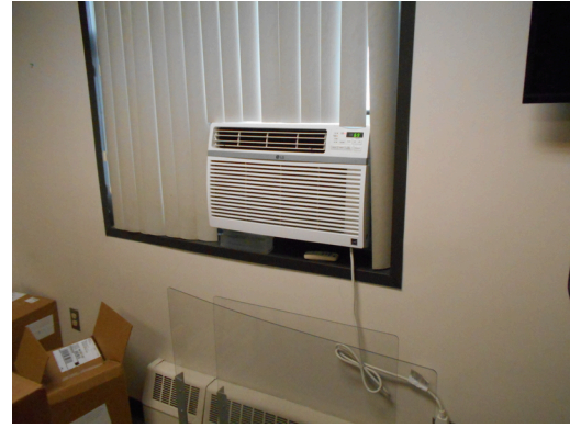
Leasing office, window mounted A/C
