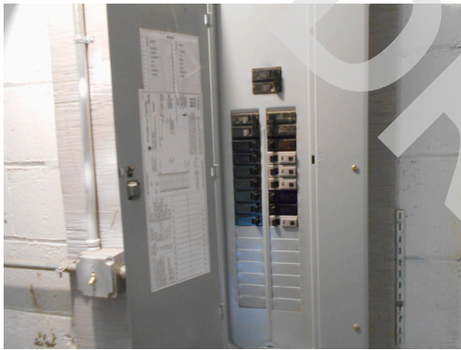
Building 3 unit 204, 28 O'Callaghan Way, 3br/1ba Townhouse - Basement electrical breaker
