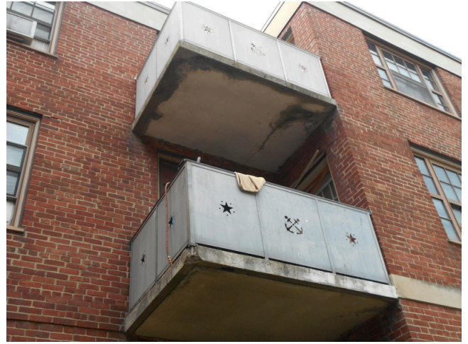
222. Building 32, concrete balcony, deterioration on underside (Critical Repair)
