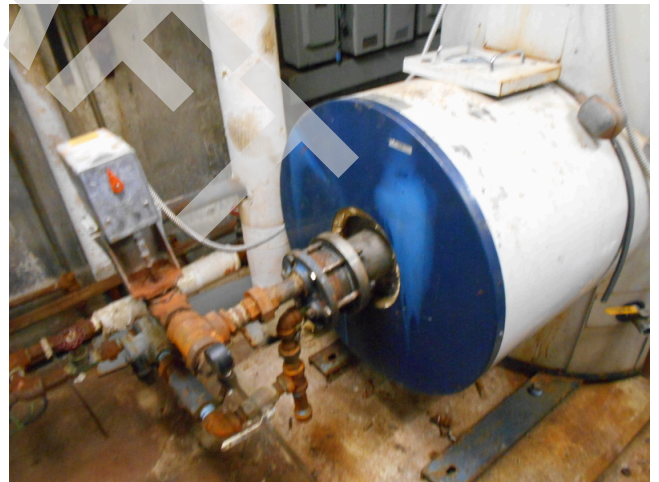
64. Building 4 mechanical room
