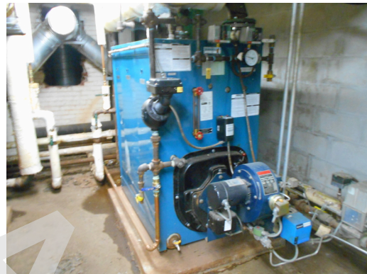
Building 32 boiler room
