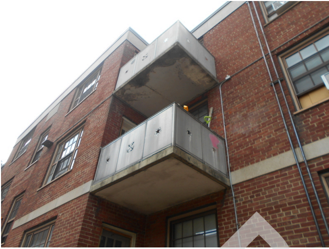
221. Building 32, concrete balcony, deterioration on underside (Critical Repair)
