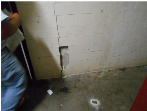
Building 23, 2 Logan Way basement, cracking CMU-wall (Non-Critical Repair)
