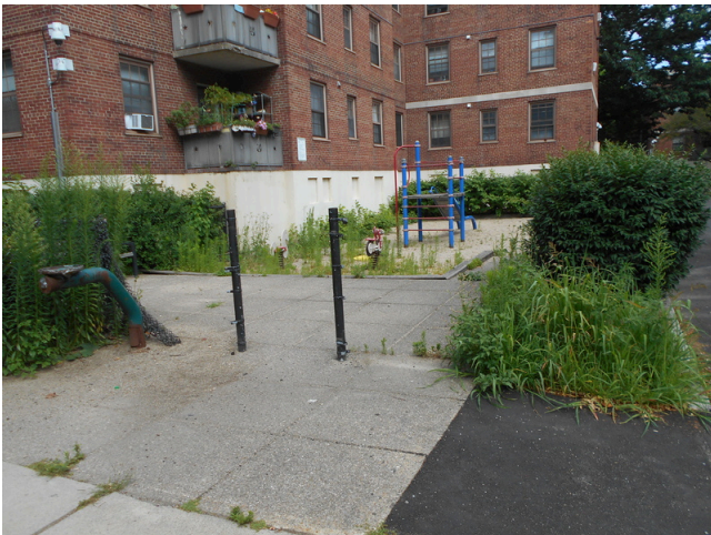
227. Playground by building 22, overgrown (Non-Critical Repair)
