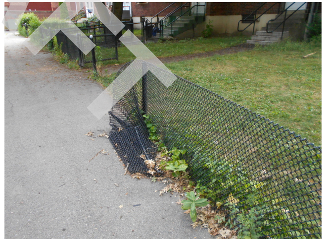
92. Damaged chain link fence by 198 O'Callaghan way, apartment 120 (Non-Critical Repair)
