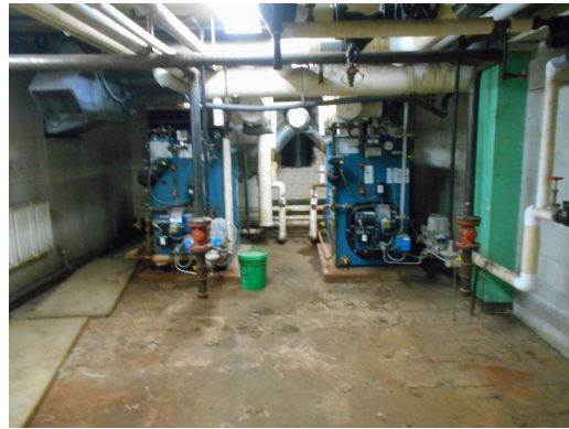
Building 32 boiler room
