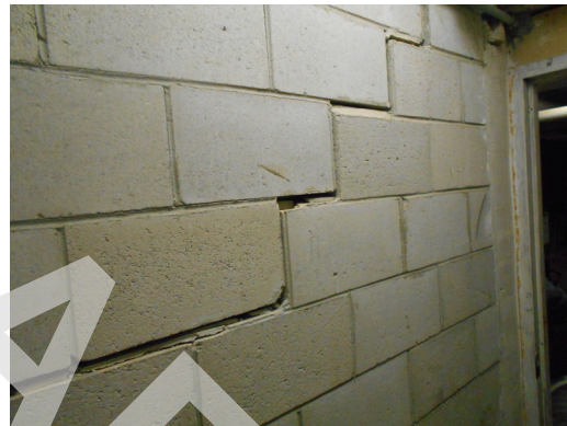
Building 30 basement, 15 Logan way, cracking CMU-wall (Non-Critical Repair)
