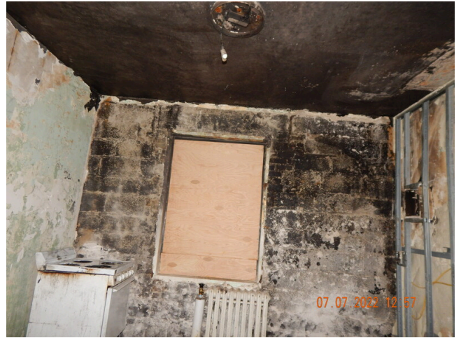
130. Units 1016 and 915 have fire damage
