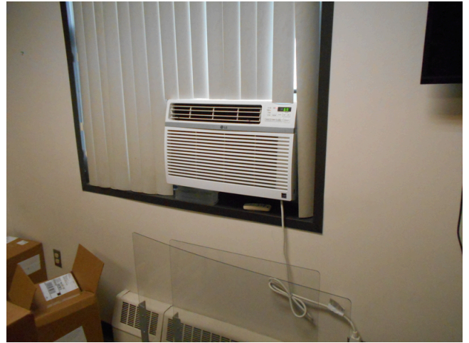
14. Leasing office, window mounted A/C
