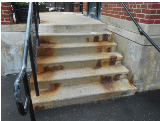
Leasing office concrete stairs, rebar rust (Non-Critical Repair)
