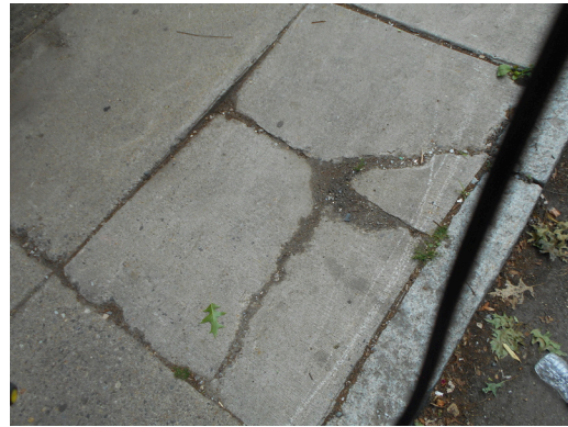
Concrete trip hazard between building 3 and building 4 (Critical Repair)
