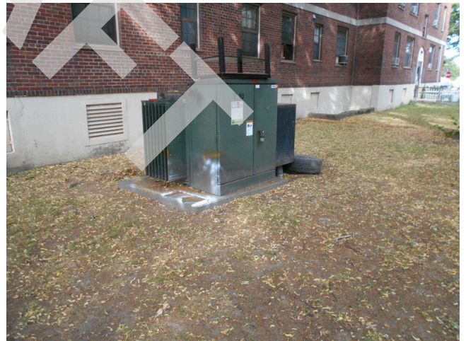
140. Pad mounted transformer
