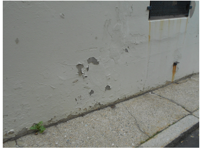
74. Paint chipping along side façade of leasing office (Non-Critical Repair)
