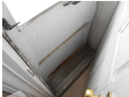
Building 5 unit 186, 64 O'Callaghan Way, 3br/1ba Townhouse - Rear door, damaged (Non-Critical Repair)
