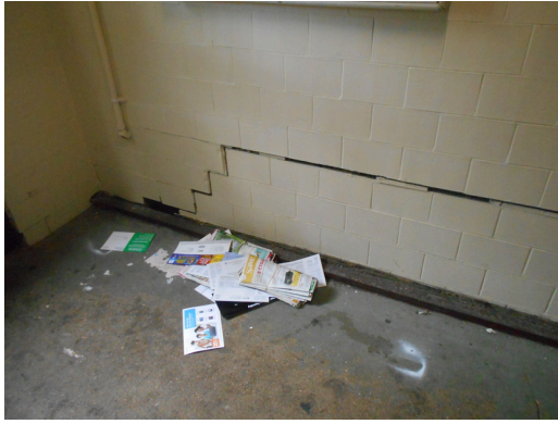
Building 17 basement, cracked (Non-Critical Repair)
