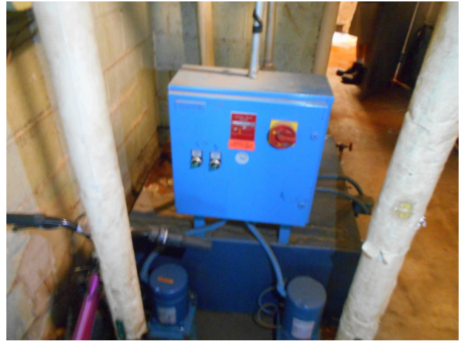
42. Leasing office boiler pump
