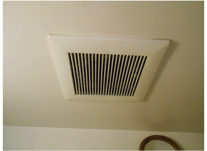
10. Building 1 unit 238, 1br/1ba - Bathroom shower, vent
