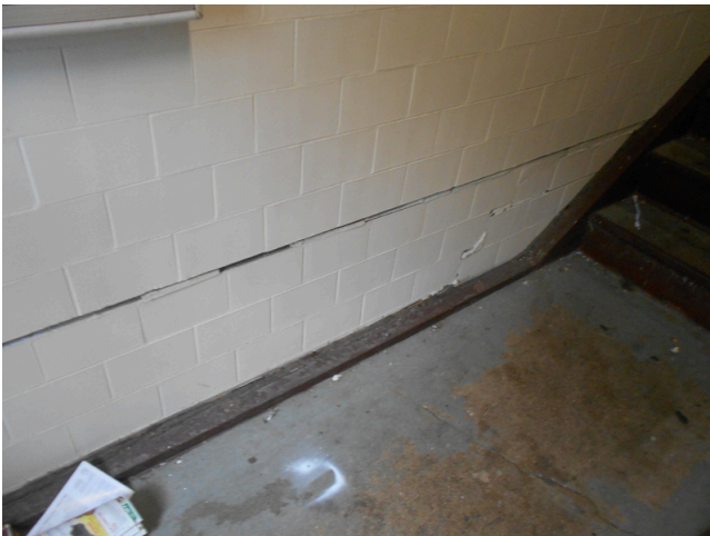
179. Building 17 basement, cracked (Non-Critical Repair)
