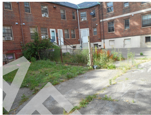
Building 4 rear façade, Cracked asphalt courtyard (Non-Critical Repair)
