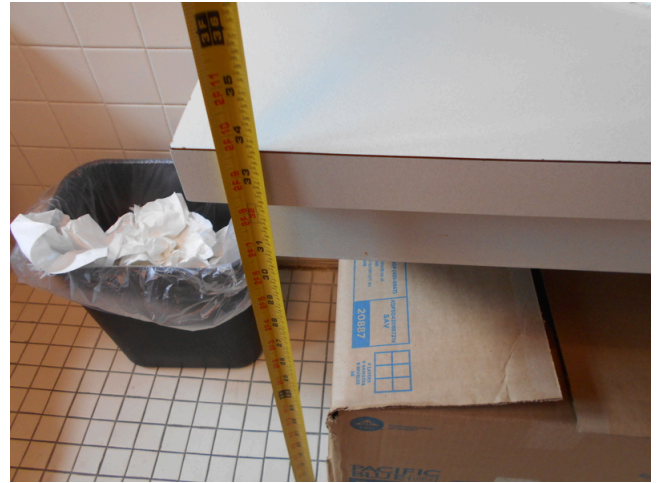
18. Leasing office public restroom sink height, 33"
