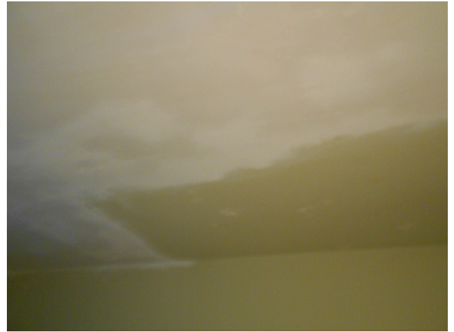
78. Building 3 unit 204, 28 O'Callaghan Way, 3br/ 1ba Townhouse - Bedroom 3, damaged paint (Non- Critical Repair)
