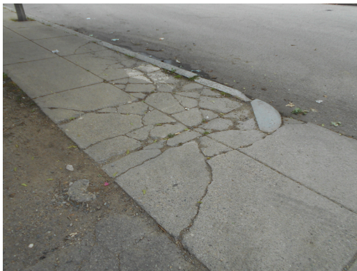
Concrete sidewalk by building 30, damaged (Critical Repair)
