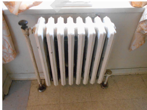
Building 4 unit 201, 34 O'Callaghan Way, 2br/1ba Townhouse - Living area/kitchen radiator
