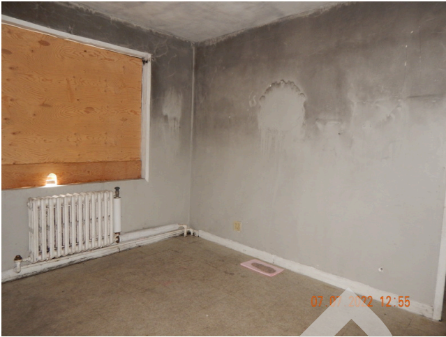
125. Units 1016 and 915 have fire damage
