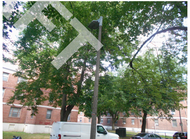
68. Typical pole mounted lighting
