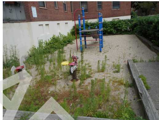
Playground by building 22, overgrown (Non-Critical Repair)
