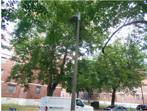
Typical pole mounted lighting
