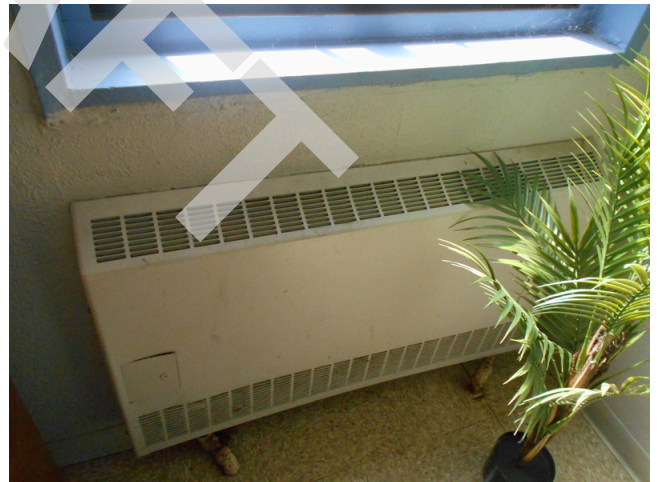
264. Community building, task force headquarters, kitchen radiator
