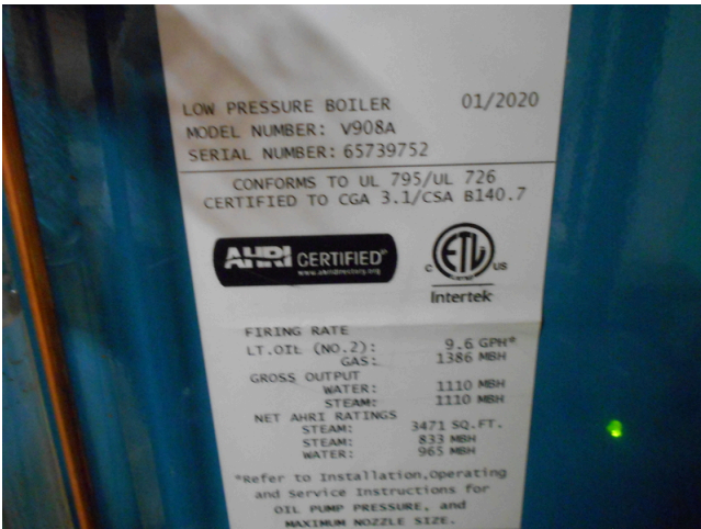
159. Building 32 boiler room
