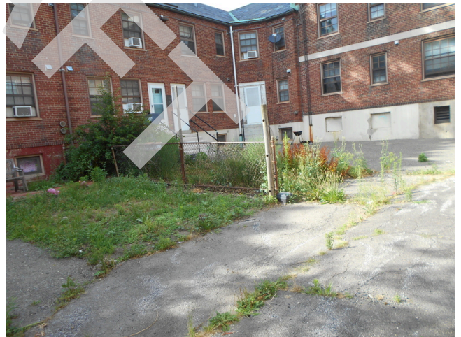
132. Building 4 rear façade, Cracked asphalt courtyard (Non-Critical Repair)
