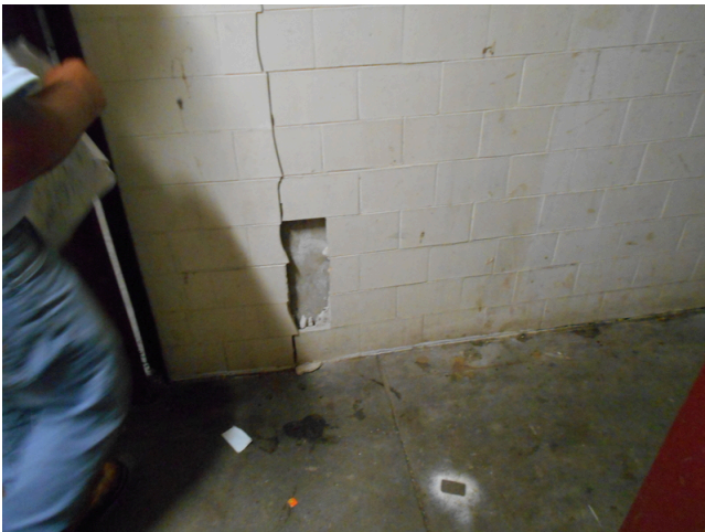
187. Building 23, 2 Logan Way basement, cracking CMU-wall (Non-Critical Repair)
