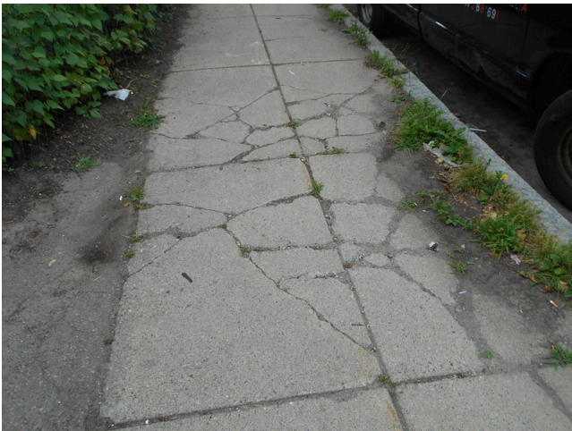
207. Concrete sidewalk by building 34, damaged (Critical Repair)
