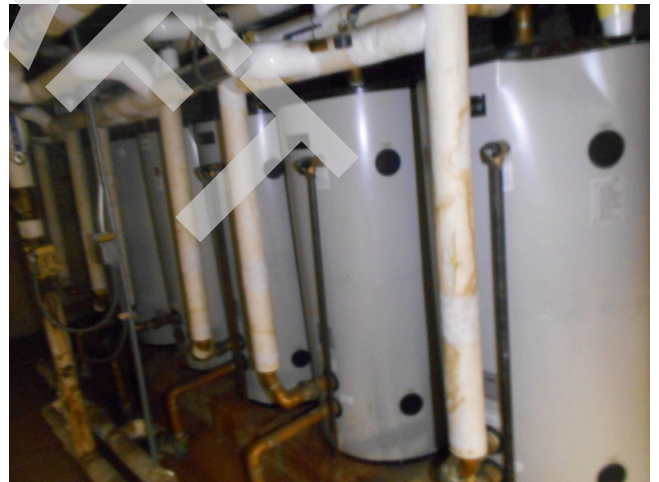
172. Building 30 basement, hot water tank
