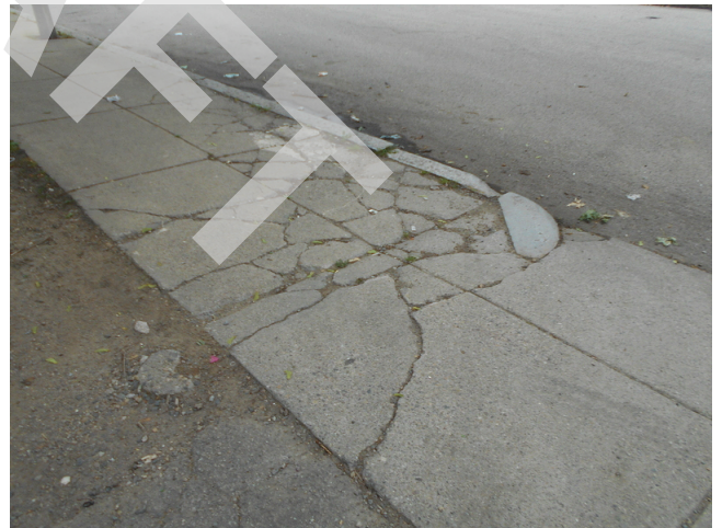
204. Concrete sidewalk by building 30, damaged (Critical Repair)
