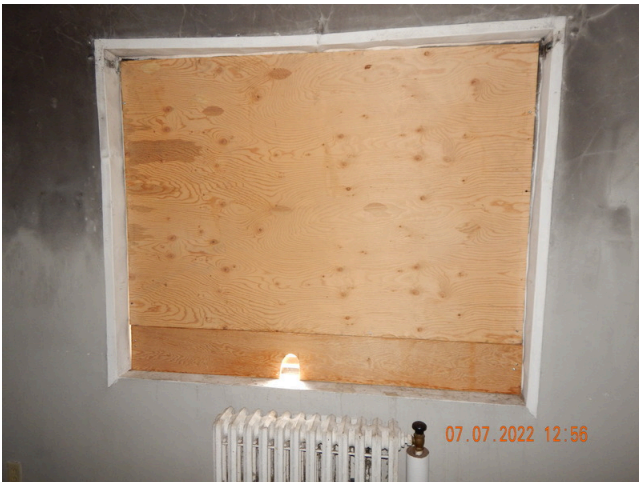
127. Units 1016 and 915 have fire damage
