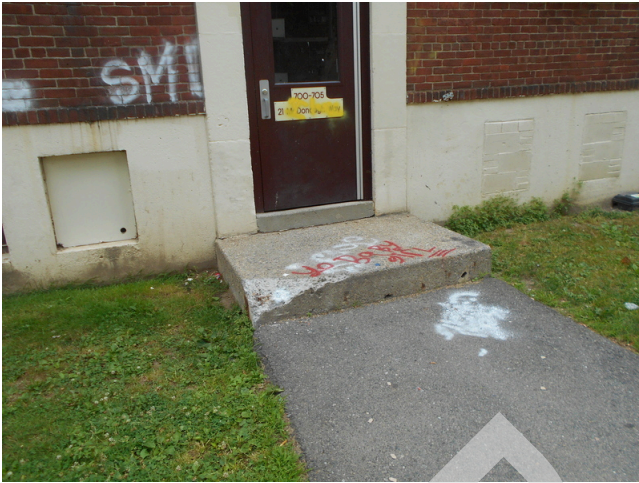
193. Building 31, 21 McDonough Way, damaged concrete pad by stairwell entrance (Non-Critical Repair)
