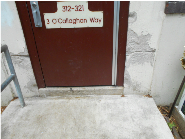
143. 3 O'Callaghan way entrance, damaged entry (Non-Critical Repair)
