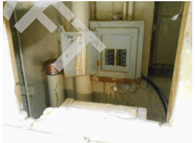
164. Building 30 basement electrical breaker
