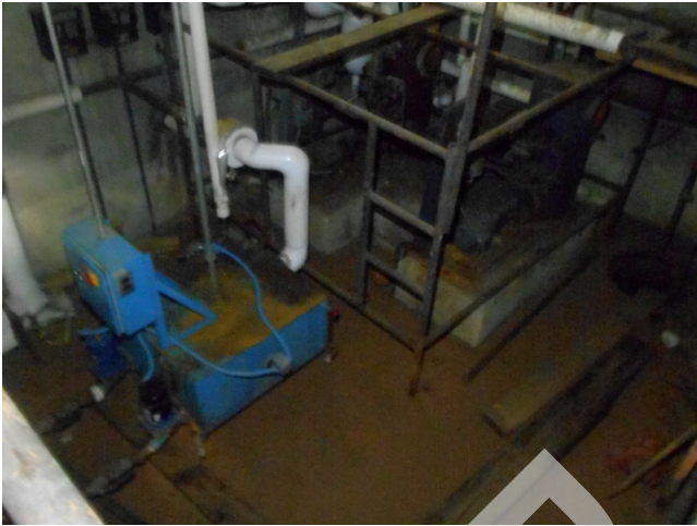
169. Building 30 basement, water pump
