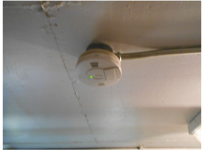
66. Building 3 unit 204, 28 O'Callaghan Way, 3br/ 1ba Townhouse - Basement smoke detector
