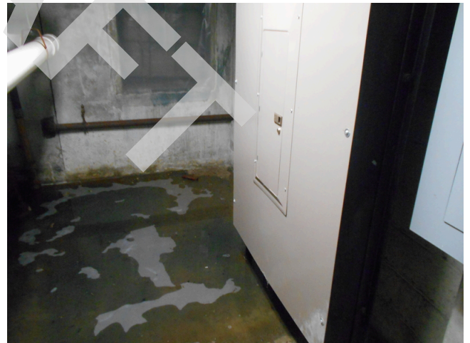
60. Building 1 basement water intrusion (Critical Repair)
