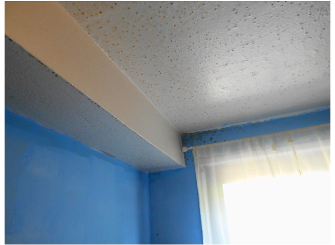
46. Building 2 unit 222, 2br/1ba - Kitchen ceiling, water damaged from uncovered stove (Non-Critical Repair)
