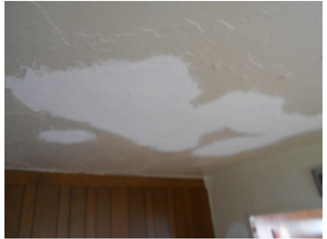
122. Building 9 unit 132, 172 O'Callaghan Way, 3br/ 1ba Townhouse - Living area, paint damaged ceiling (Non-Critical Repair)
