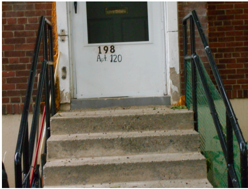
Building 11 front façade, chipping paint on door of 198 O'Callaghan Way, Apartment 120 (Non-Critical Repair)
