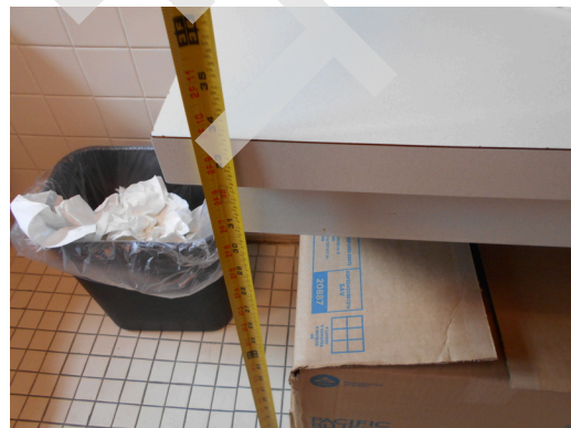
Leasing office public restroom sink height, 33"
