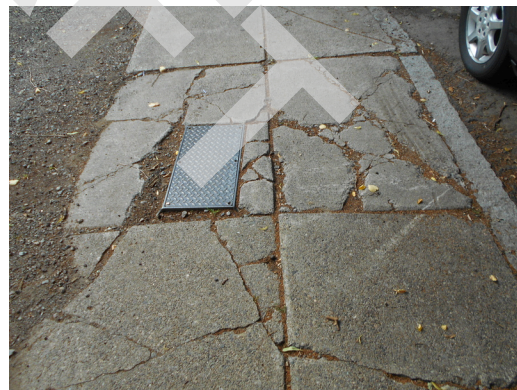
Concrete sidewalk by building 7, damaged (Critical Repair)
