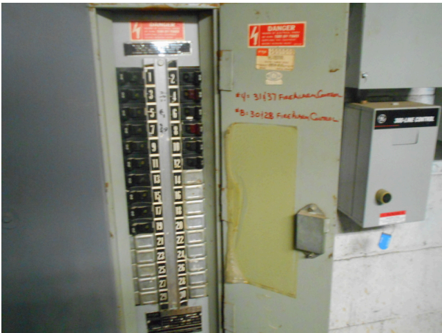
175. Building 30 electrical panel, federal pacific (Non-Critical Repair)
