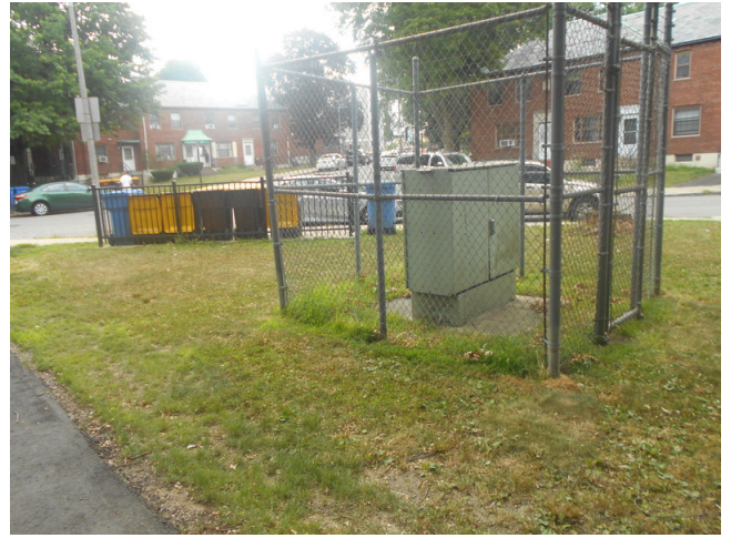
242. Pad mounted electrical transformer
