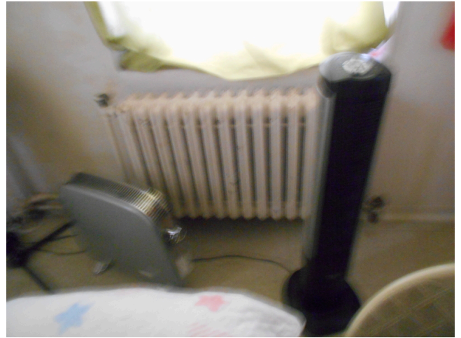
18. Building 1 unit 238, 1br/1ba - Bedroom radiator
