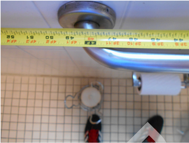
25. Leasing office public restroom side grab bar, 48" (Critical Repair)
