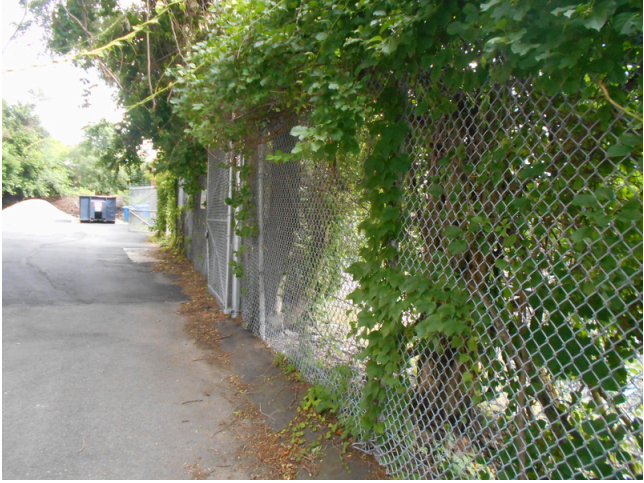
82. Chain link fence along leasing office driveway, overgrown
