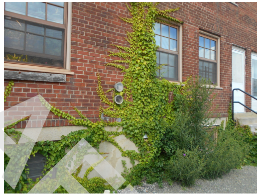
Building 5 rear façade, foliage growing along façade (Non-Critical Repair)
