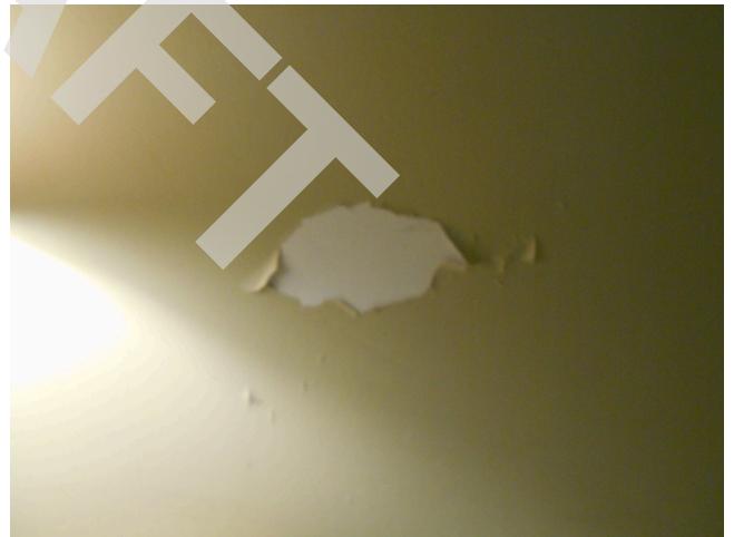
76. Building 3 unit 204, 28 O'Callaghan Way, 3br/ 1ba Townhouse - Bedroom 2, damaged paint (Non- Critical Repair)
