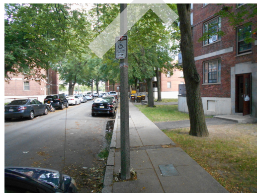
Building 3 handicap street parking, no curb cut or access aisle (Critical Repair)
