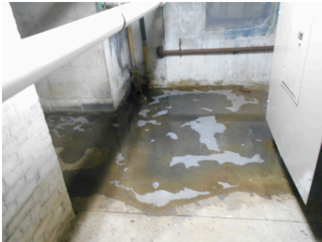
59. Building 1 basement water intrusion (Non-Critical Repair)
