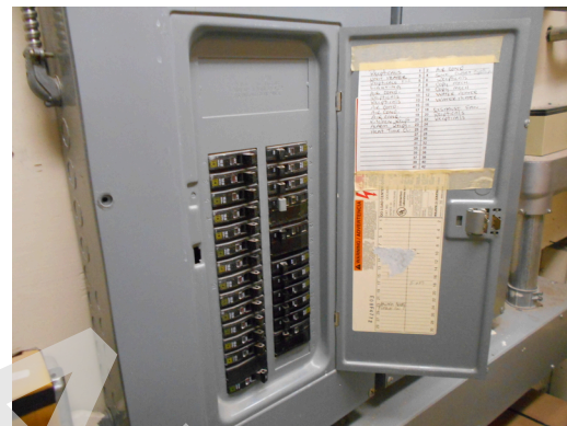
Leasing office electrical panel
