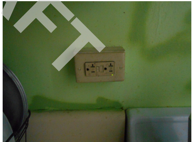
16. Building 1 unit 238, 1br/1ba - Kitchen GFCI
