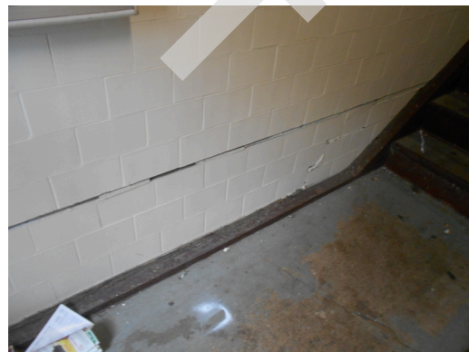
Building 17 basement, cracked (Non-Critical Repair)
