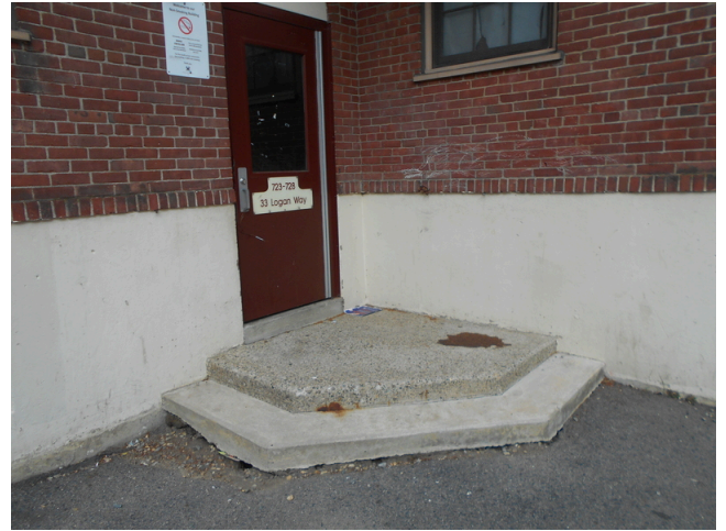
214. Building 32, 33 Logan way stairwell entrance, Concrete stairs at entrance eroded (Non-Critical Repair)
