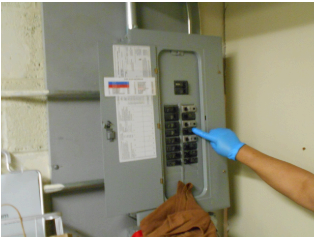
115. Building 5 unit 186, 64 O'Callaghan Way, 3br/ 1ba Townhouse - Basement electrical breaker
