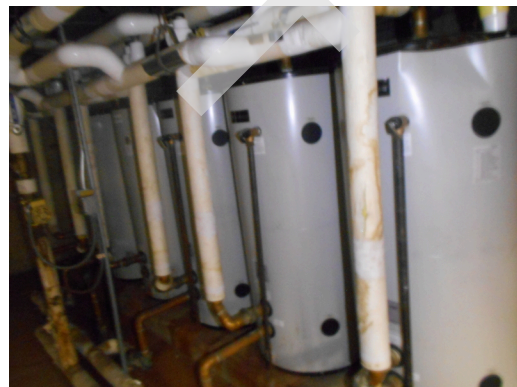
Building 30 basement, hot water tank
