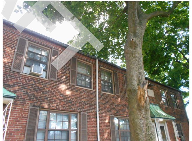
128. Building 3 front façade, trees growing along side building (Non-Critical Repair)
