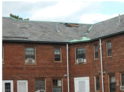
Building 3 rear façade, damaged slate tile roofing (Non-Critical Repair)
