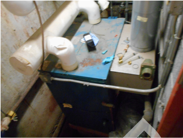
41. Leasing office boiler
