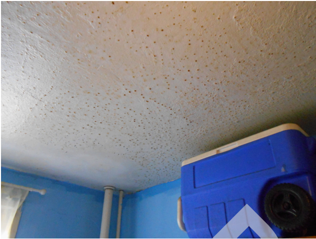
45. Building 2 unit 222, 2br/1ba - Kitchen ceiling, water damaged from uncovered stove (Non-Critical Repair)
