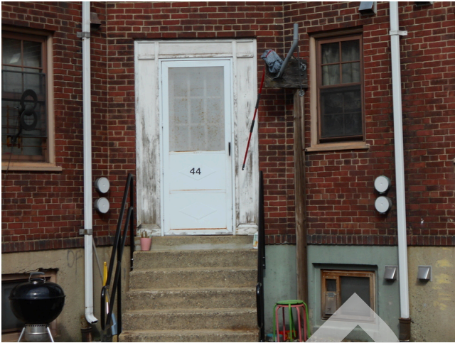
237. Paint chipping along rear entrance of unit 44 O'Callaghan way, unit 196 (Non-Critical Repair)
