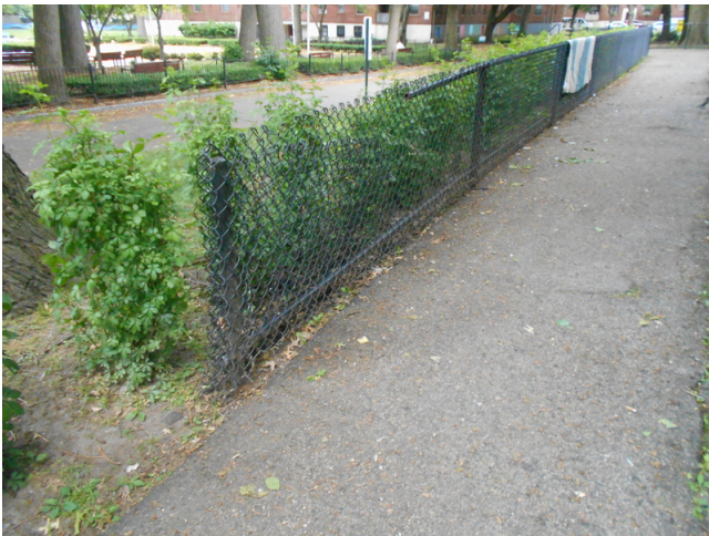
235. Damaged chain link fence by Sterling square drive (Non-Critical Repair)
