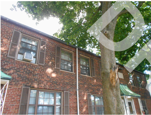
Building 3 front façade, trees growing along side building (Non-Critical Repair)
