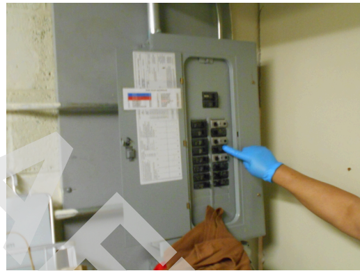
Building 5 unit 186, 64 O'Callaghan Way, 3br/1ba Townhouse - Basement electrical breaker
