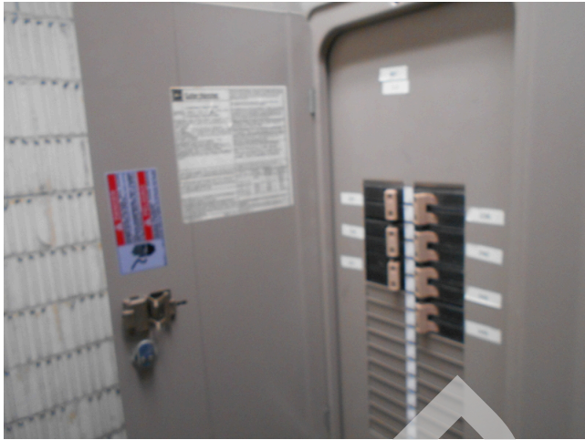
57. Building 1 basement electrical panel
