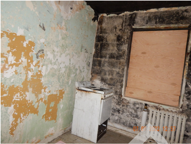
129. Units 1016 and 915 have fire damage
