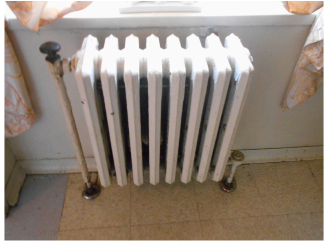
82. Building 4 unit 201, 34 O'Callaghan Way, 2br/ 1ba Townhouse - Living area/kitchen radiator
