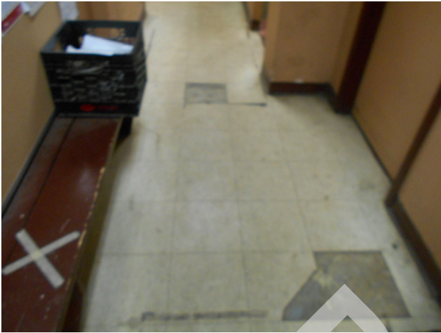
37. Leasing office basement, damaged vinyl tile (Non-Critical Repair)
