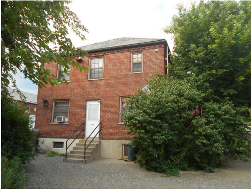
Building 4 side façade, foliage growing along building façade (Non-Critical Repair)
