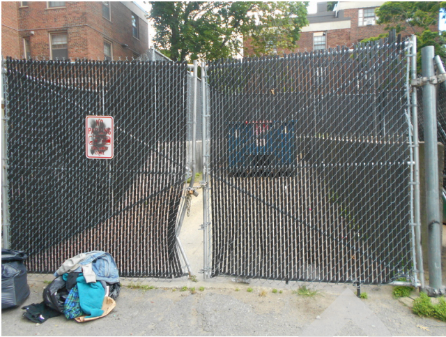
197. Refuse area by building 30, damaged fencing (Non-Critical Repair)
