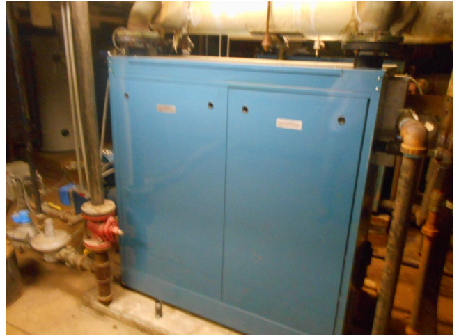
170. Building 30 basement, boiler
