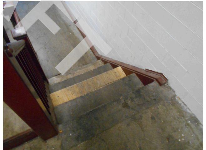
184. Building 19, 2 Sterling square stairwell, damaged stairs (Non-Critical Repair)
