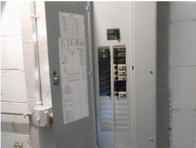
67. Building 3 unit 204, 28 O'Callaghan Way, 3br/ 1ba Townhouse - Basement electrical breaker
