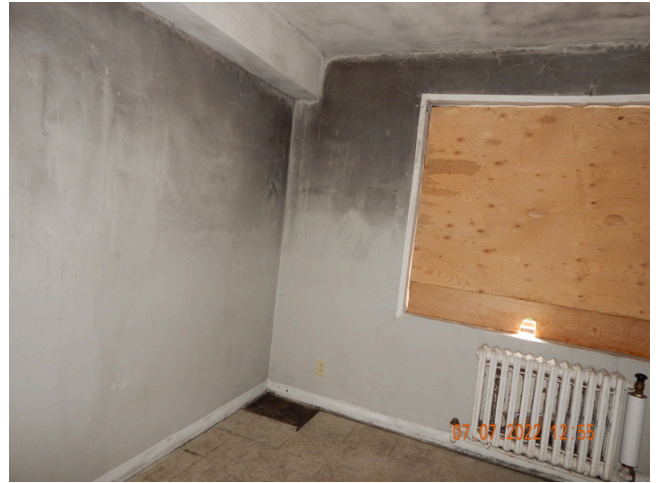
126. Units 1016 and 915 have fire damage
