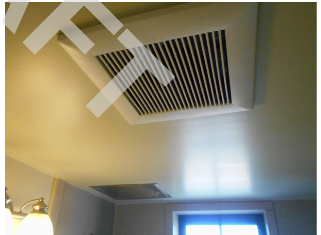
32. Building 1 unit 247, 1br/1ba - Bathroom ceiling
