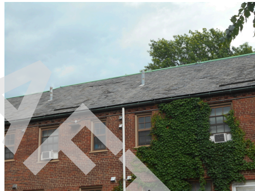
Building 6 slate tile roofing, shingles falling (Non-Critical Repair)
