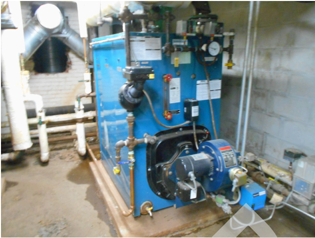
157. Building 32 boiler room
