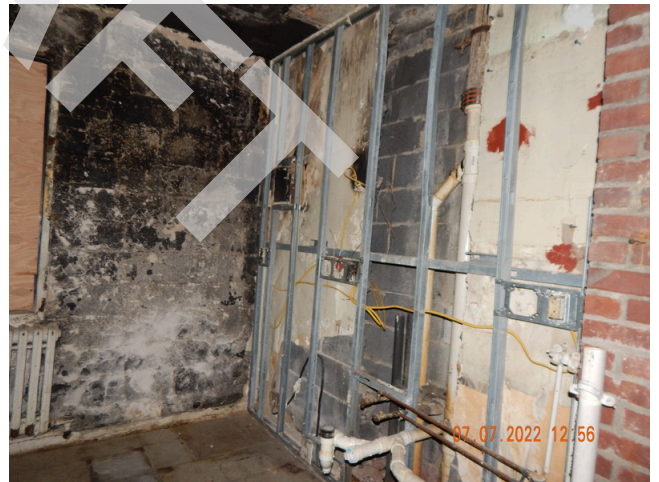
128. Units 1016 and 915 have fire damage
