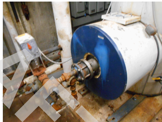
Building 4 mechanical room
