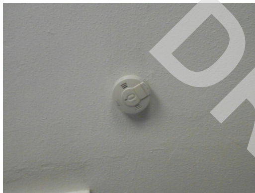
Community building, task force headquarters, smoke detector
