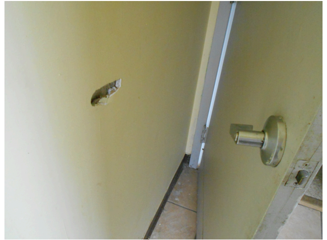
282. Community building, task force headquarters, restroom 2 drywall damaged by door handle (Non-Critical Repair)
