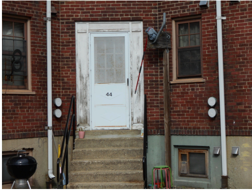
Paint chipping along rear entrance of unit 44 O'Callaghan way, unit 196 (Non-Critical Repair)
