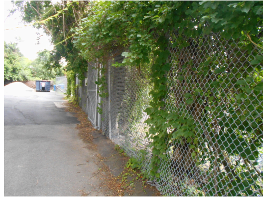
Chain link fence along leasing office driveway, overgrown
