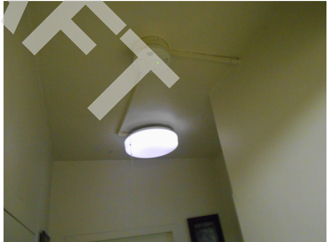
4. Building 1 unit 238, 1br/1ba - Living area smoke detector
