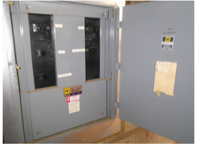
62. Building 1 electrical main
