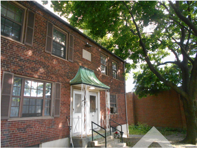
129. Building 3 side façade, trees growing along side building (Non-Critical Repair)
