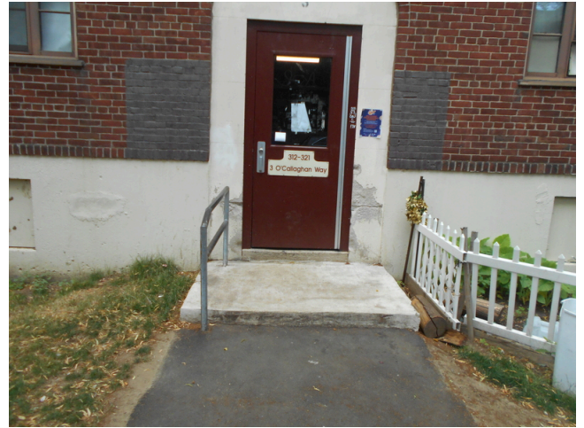
142. 3 O'Callaghan way entrance, damaged entry (Non-Critical Repair)
