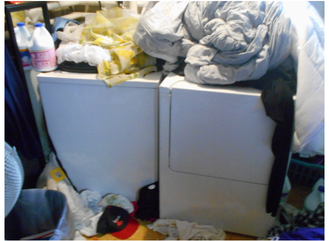
90. Building 4 unit 201, 34 O'Callaghan Way, 2br/ 1ba Townhouse - Basement electrical Washer/dryers
