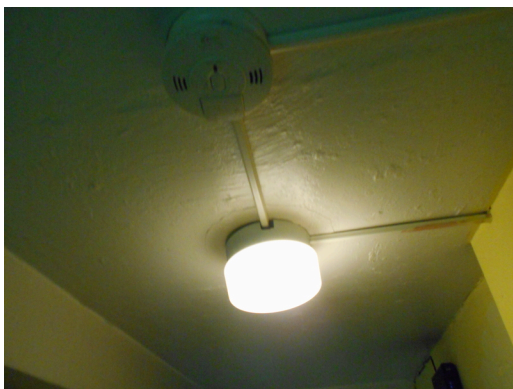
Building 2 unit 222, 2br/1ba - Living area smoke detector
