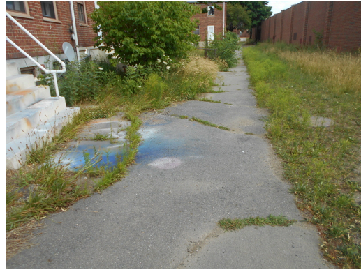
Building 3 rear façade, asphalt pathway overgrown and cracked (Non-Critical Repair)
