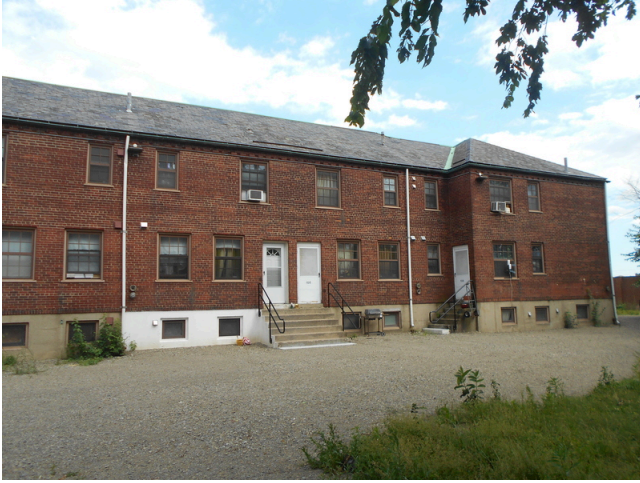
98. Building 6 rear façade, poor condition shingles (Non-Critical Repair)
