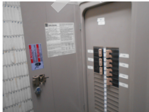
Building 1 basement electrical panel
