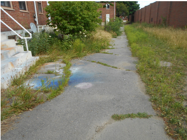
127. Building 3 rear façade, asphalt pathway overgrown and cracked (Non-Critical Repair)
