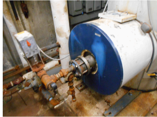
Building 4 mechanical room
