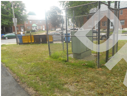
Pad mounted electrical transformer
