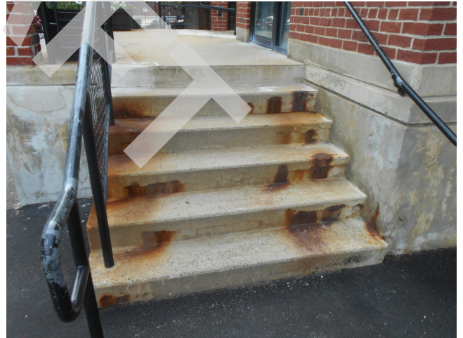
12. Leasing office concrete stairs, rebar rust (Non-Critical Repair)
