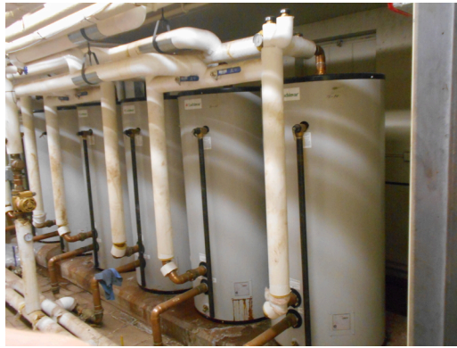
Building 32 boiler room hot water tanks
