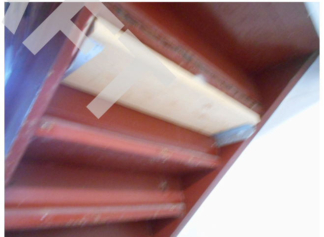
148. Building 32, 41 Logan way stairwell, damaged stairs (Non-Critical Repair)
