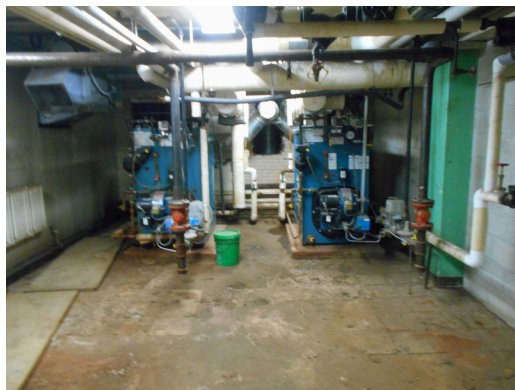
Building 32 boiler room
