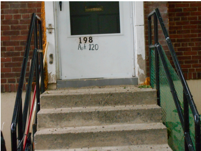
91. Building 11 front façade, chipping paint on door of 198 O'Callaghan Way, Apartment 120 (Non-Critical Repair)
