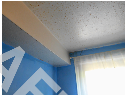
Building 2 unit 222, 2br/1ba - Kitchen ceiling, water damaged from uncovered stove (Non-Critical Repair)
