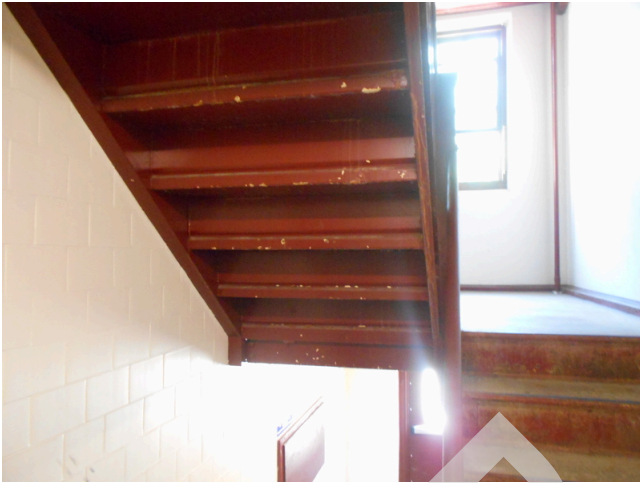
53. Typical stairwell, paint chipping (Non-Critical Repair)
