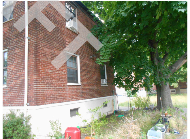
120. Building 3 rear façade, foliage growing along building façade (Non-Critical Repair)
