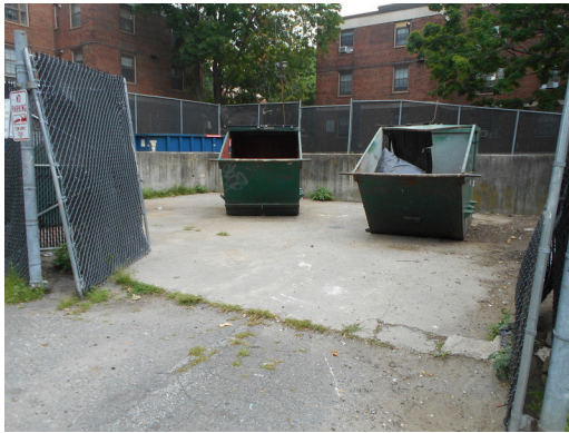
Refuse area by building 30, damaged fencing (Non-Critical Repair)
