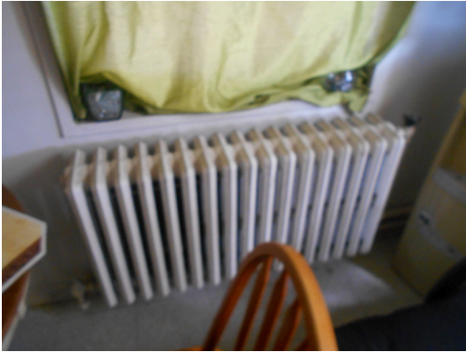
Building 1 unit 238, 1br/1ba - Living area steam radiator
