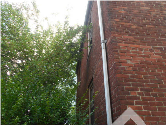
109. Building 5 side façade, foliage growing along building façade (Non-Critical Repair)
