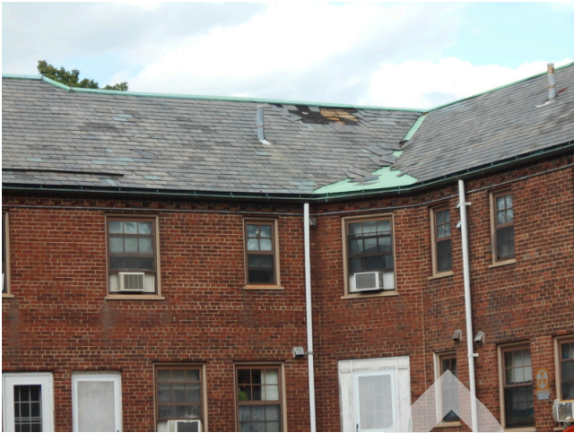
125. Building 3 rear façade, damaged slate tile roofing (Non-Critical Repair)
