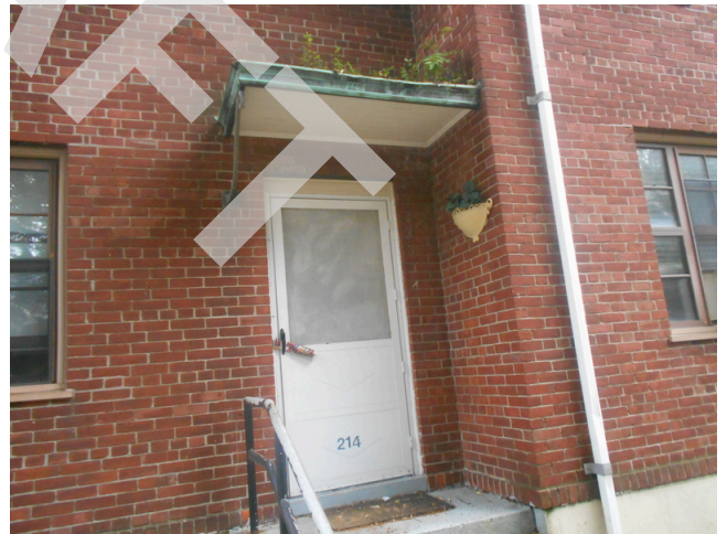
236. Plants growing on awning of 214 O'Callaghan Way, unit 113 (Non-Critical Repair)
