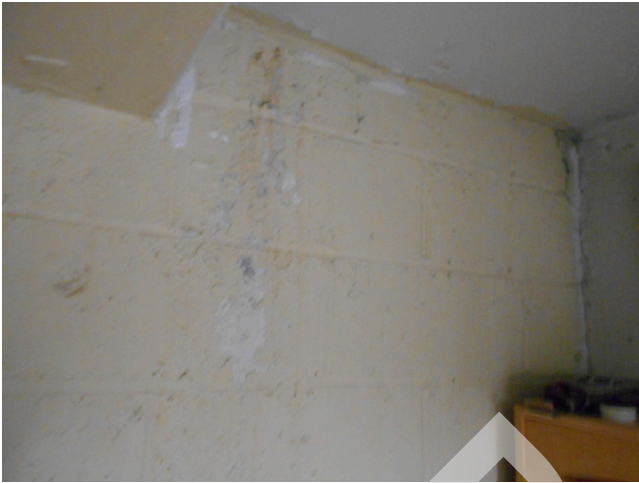
69. Building 3 unit 204, 28 O'Callaghan Way, 3br/ 1ba Townhouse - Basement paint damaged
