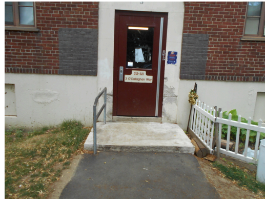
3 O'Callaghan way entrance, damaged entry (Non-Critical Repair)
