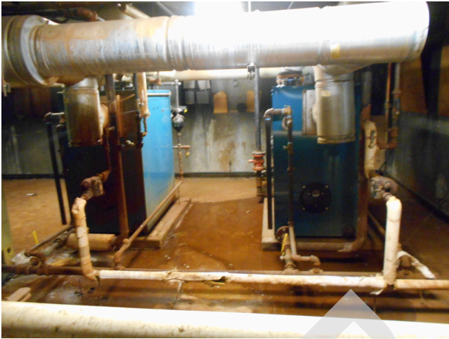
177. Building 17 basement boiler room, water pooling (Non-Critical Repair)
