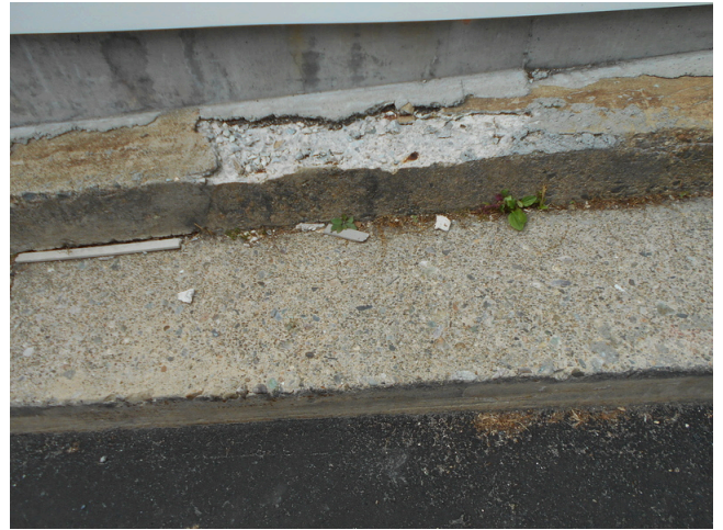
78. Leasing office side façade, damaged concrete (Non-Critical Repair)
