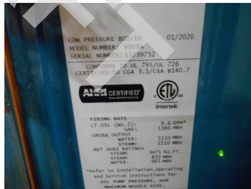
Building 32 boiler room
