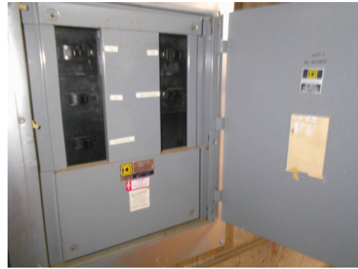
Building 1 electrical main
