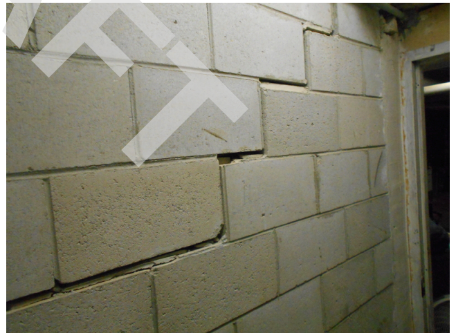
168. Building 30 basement, 15 Logan way, cracking CMU-wall (Non-Critical Repair)
