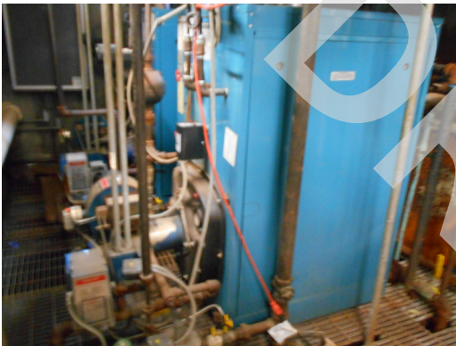
Building 4 mechanical room boilers
