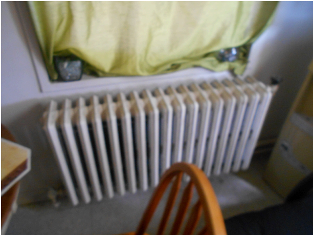
3. Building 1 unit 238, 1br/1ba - Living area steam radiator
