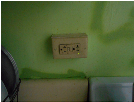
Building 1 unit 238, 1br/1ba - Kitchen GFCI
