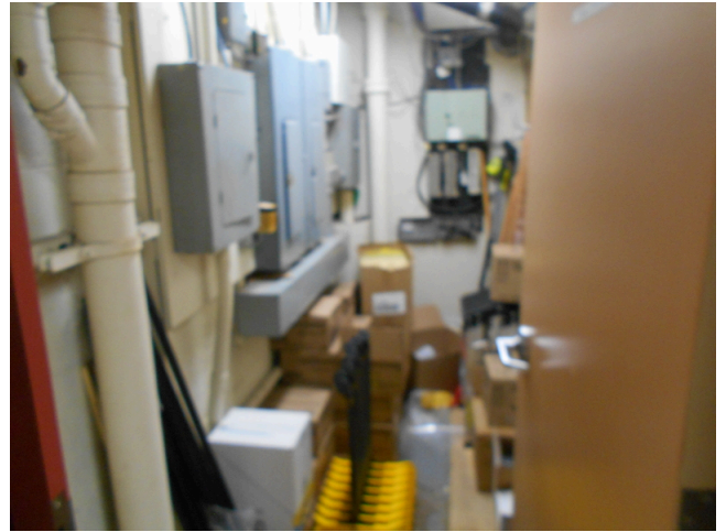
38. Leasing office electrical room, remove debris from the room (Critical Repair)
