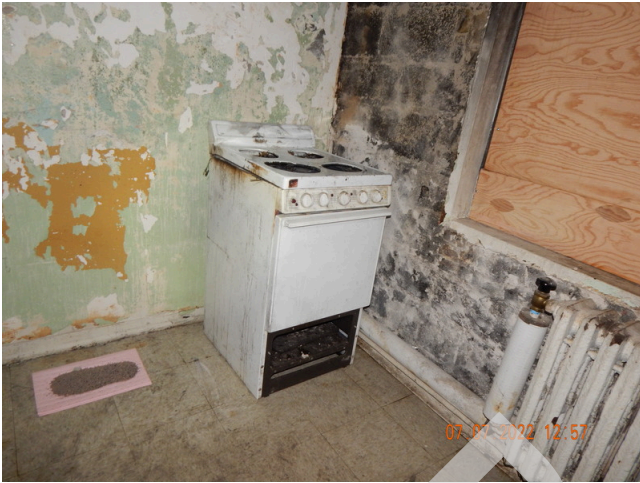
133. Units 1016 and 915 have fire damage
