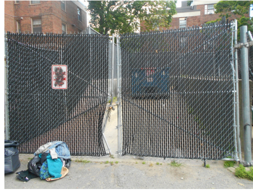
Refuse area by building 30, damaged fencing (Non-Critical Repair)
