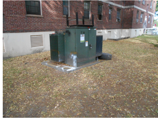
Pad mounted transformer
