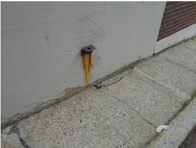
75. Paint chipping along side façade of leasing office (Non-Critical Repair)
