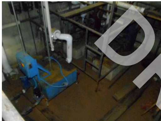
Building 30 basement, water pump
