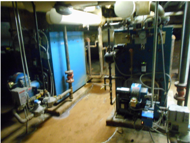
171. Building 30 basement, boiler
