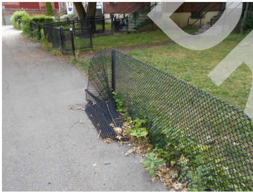
Damaged chain link fence by 198 O'Callaghan way, apartment 120 (Non-Critical Repair)
