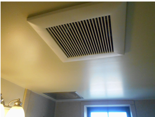
Building 1 unit 247, 1br/1ba - Bathroom ceiling
