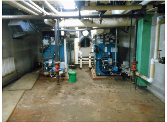
158. Building 32 boiler room
