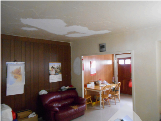
121. Building 9 unit 132, 172 O'Callaghan Way, 3br/ 1ba Townhouse - Living area, paint damaged ceiling (Non-Critical Repair)
