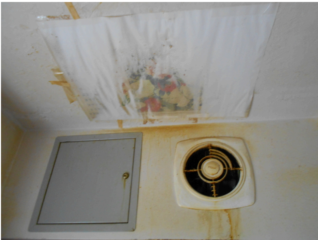
123. Building 9 unit 132, 172 O'Callaghan Way, 3br/ 1ba Townhouse - Kitchen, water damaged ceiling (Non-Critical Repair)
