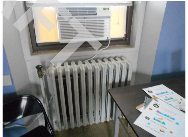
276. Community building, task force headquarters, A/C unit and radiator
