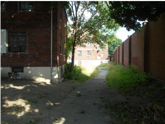
131. Building 4 side façade, trees growing along side building (Non-Critical Repair)
