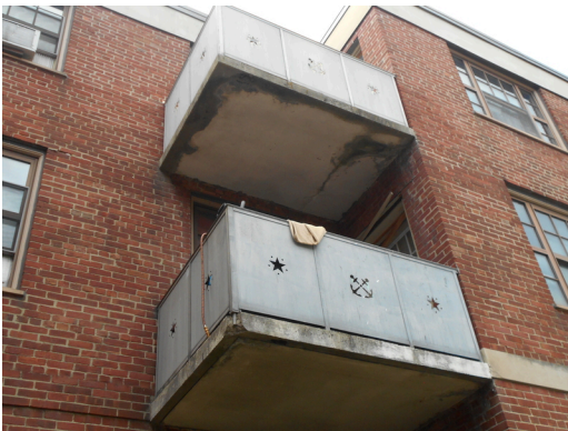
Building 32, concrete balcony, deterioration on underside (Critical Repair)
