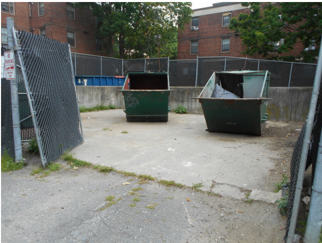
195. Refuse area by building 30, damaged fencing (Non-Critical Repair)
