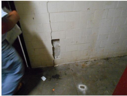
Building 23, 2 Logan Way basement, cracking CMU-wall (Non-Critical Repair)
