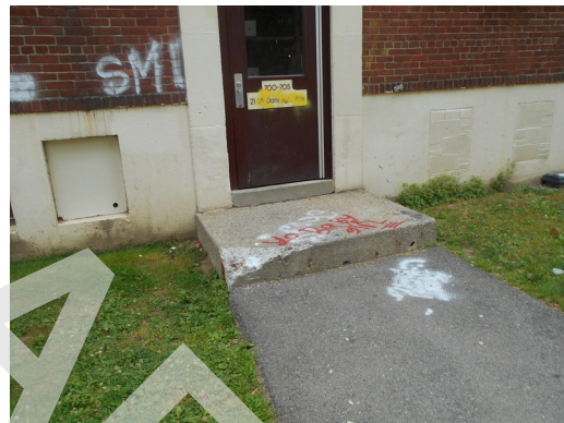
Building 31, 21 McDonough Way, damaged concrete pad by stairwell entrance (Non-Critical Repair)
