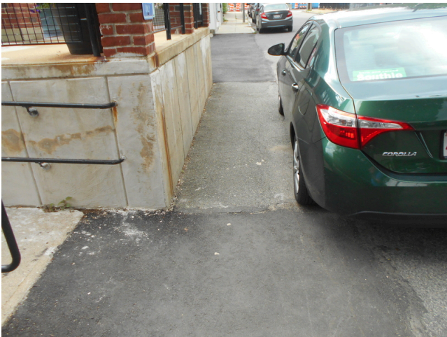
71. Leasing office accessible parking space sign, no parking space markings, no access aisle, no horizontal signage (Critical Repair)
