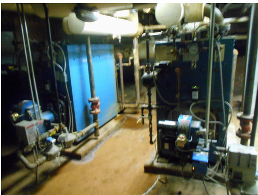
Building 30 basement, boiler
