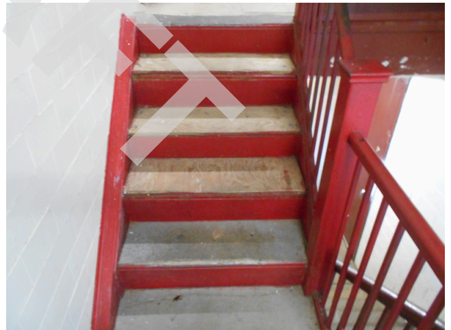
156. Building 32, 37 Logan way stairwell, damaged stairs (Non-Critical Repair)
