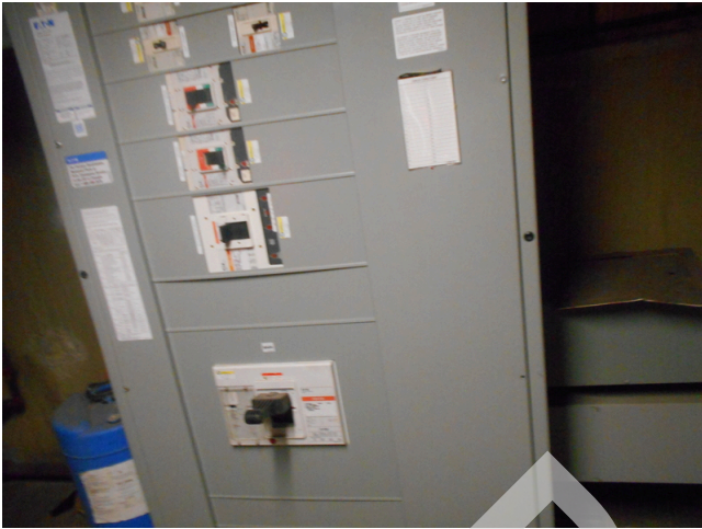
173. Building 30 electrical main
