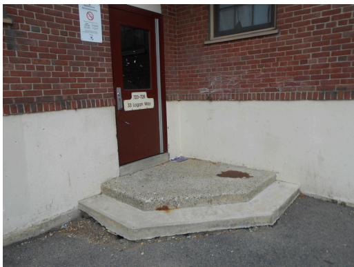
Building 32, 33 Logan way stairwell entrance, Concrete stairs at entrance eroded (Non-Critical Repair)
