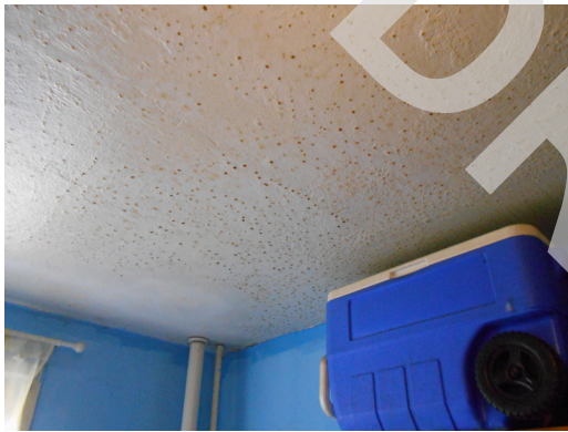
Building 2 unit 222, 2br/1ba - Kitchen ceiling, water damaged from uncovered stove (Non-Critical Repair)
