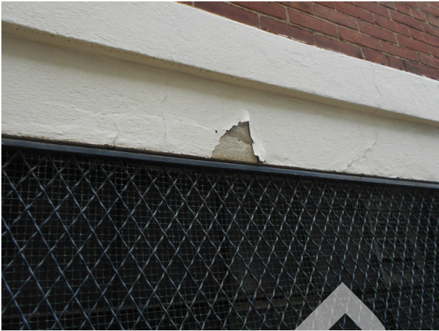
77. Paint chipping along side façade of leasing office (Non-Critical Repair)
