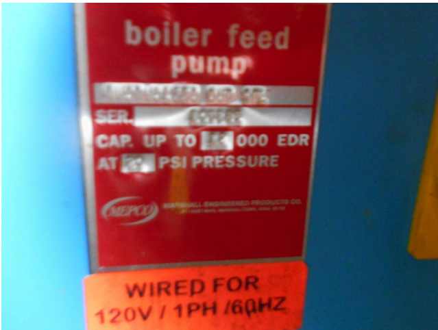
43. Leasing office boiler pump
