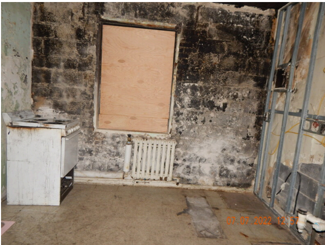
131. Units 1016 and 915 have fire damage
