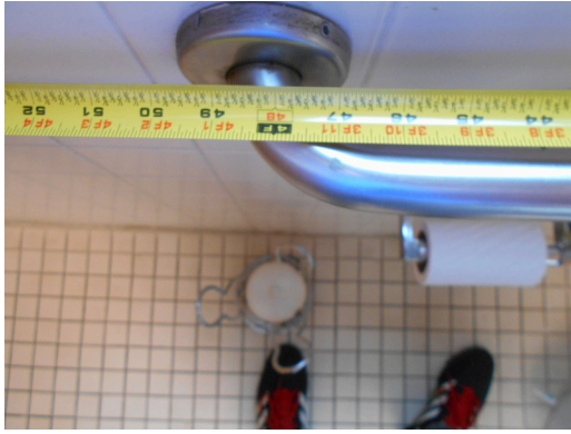
Leasing office public restroom side grab bar, 48" (Critical Repair)
