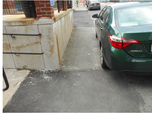
Leasing office accessible parking space sign, no parking space markings, no access aisle, no horizontal signage (Critical Repair)
