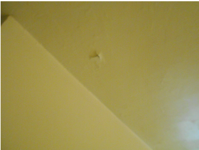
75. Building 3 unit 204, 28 O'Callaghan Way, 3br/ 1ba Townhouse - Bedroom 2, damaged paint (Non- Critical Repair)
