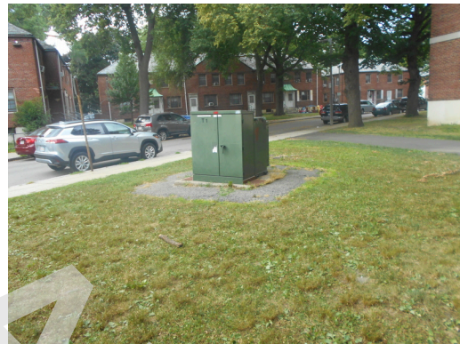
Pad mounted electrical transformer
