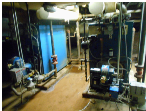
Building 30 basement, boiler
