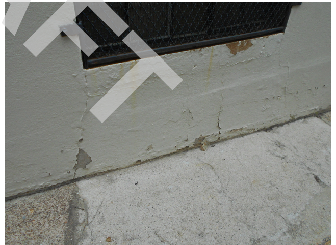
76. Paint chipping along side façade of leasing office (Non-Critical Repair)
