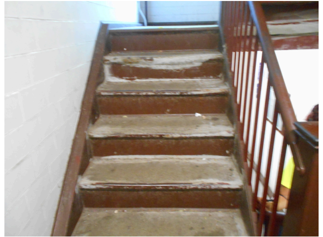
54. Typical stairwell, stairs damaged (Non-Critical Repair)
