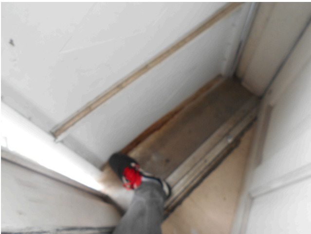
119. Building 5 unit 186, 64 O'Callaghan Way, 3br/1ba Townhouse - Rear door, damaged (Non-Critical Repair)
