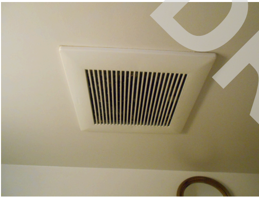
Building 1 unit 238, 1br/1ba - Bathroom shower, vent
