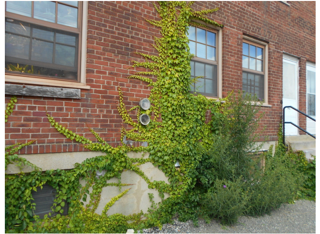
106. Building 5 rear façade, foliage growing along façade (Non-Critical Repair)
