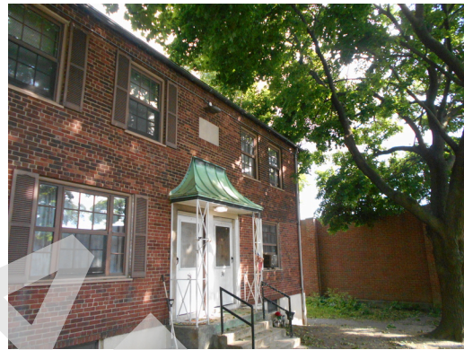
Building 3 side façade, trees growing along side building (Non-Critical Repair)
