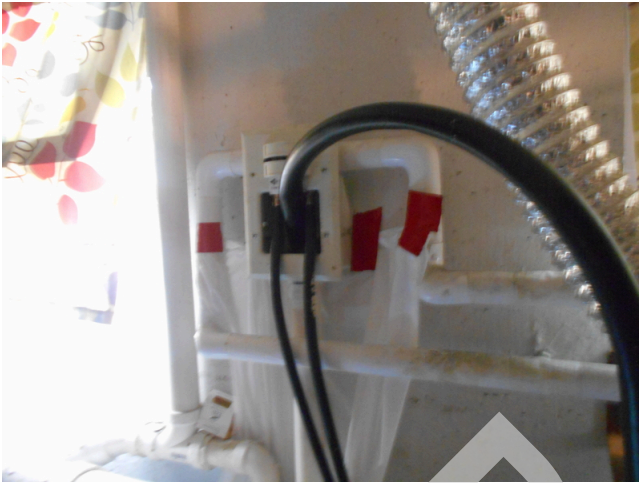
65. Building 3 unit 204, 28 O'Callaghan Way, 3br/ 1ba Townhouse - Basement laundry hook-up
