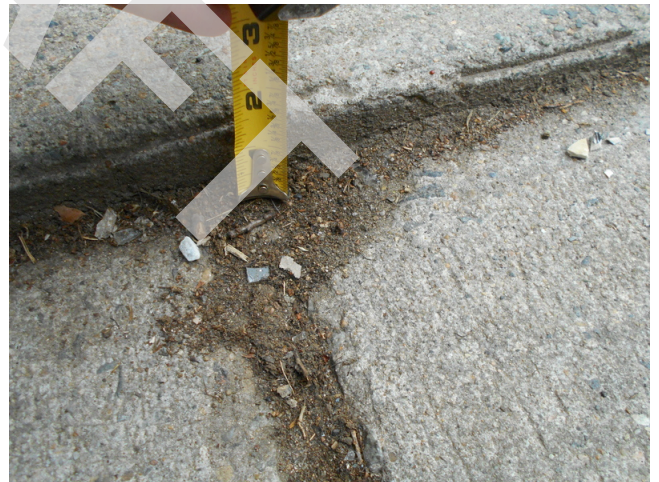
116. Concrete trip hazard between building 3 and building 4 (Critical Repair)
