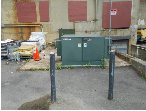
Pad mounted electrical transformers
