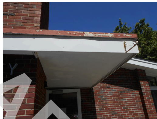
Community building, paint chipping (Non-Critical Repair)
