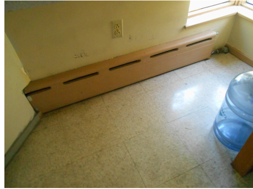
Community building steam radiator
