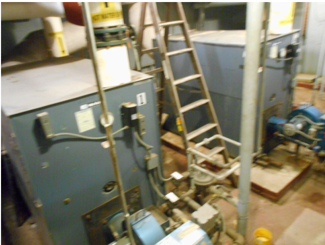
55. Basement mechanical room, heating boilers
