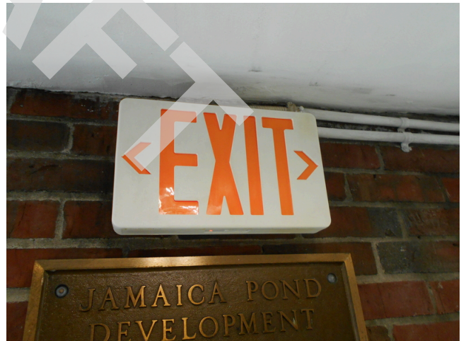
108. Emergency exit sign
