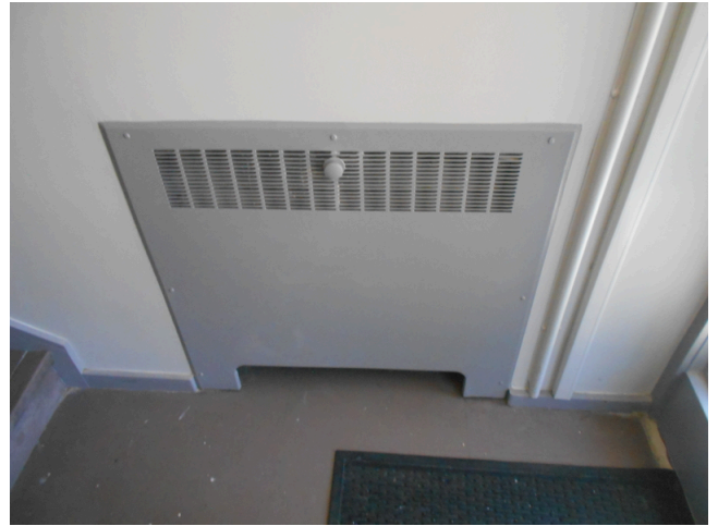
102. Typical stairwell entrance radiator
