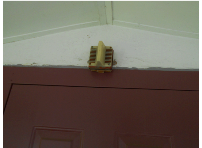
118. Typical emergency pull cord light above stairwell entrances
