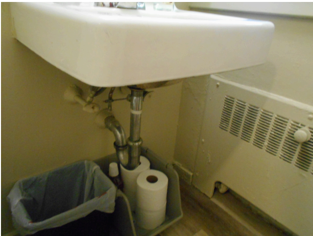
11. Building A, Unit 9, 1br/1ba - Bathroom sink, no scald abrasion protection
