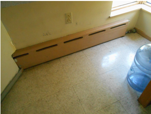
43. Community building steam radiator
