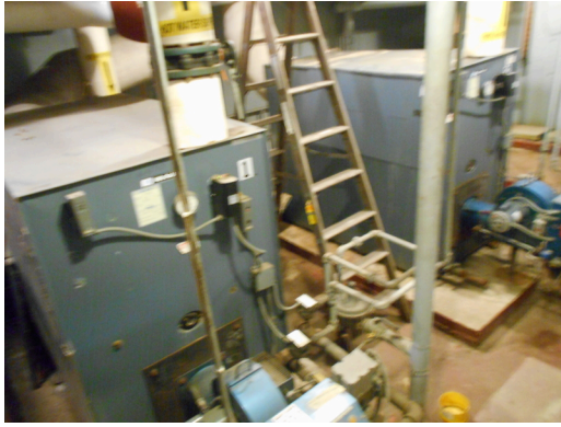
Basement mechanical room, heating boilers
