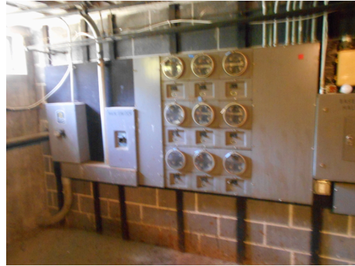
Building B basement electric meters
