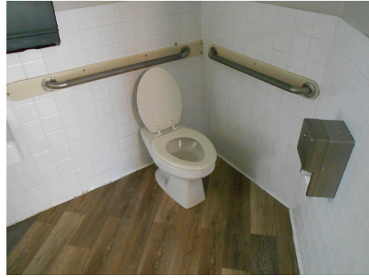
Men's public restroom, not enough clear floor space (Critical Repair)
