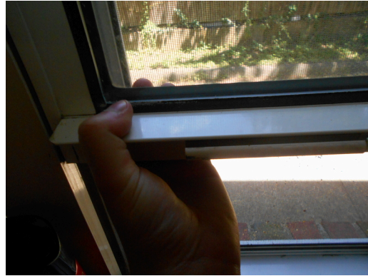
Building A, Unit 9, 1br/1ba - Typical window
