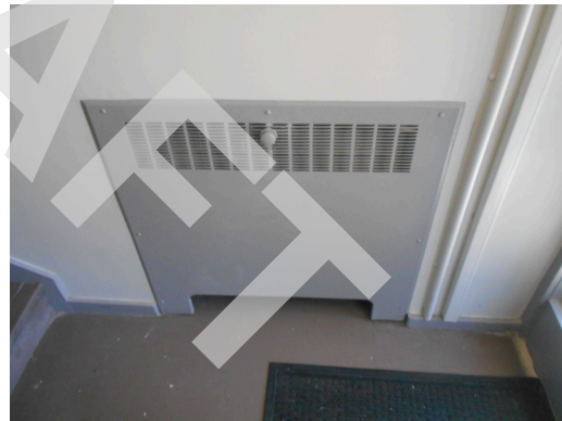
Typical stairwell entrance radiator
