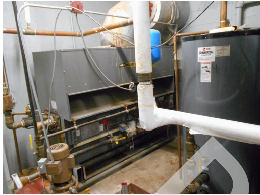
Basement mechanical room, water heater
