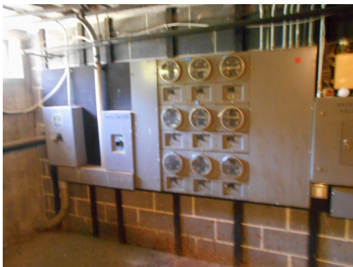
Building B basement electric meters
