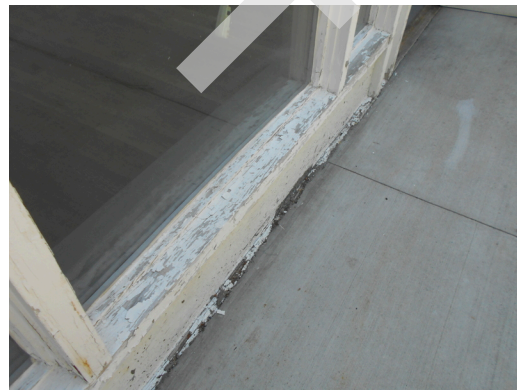
Community building rear façade, paint chipping (Non-Critical Repair)
