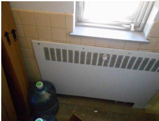
Community building steam radiator
