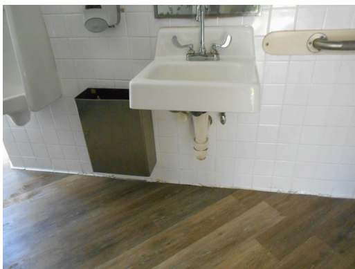
Men's public restroom, no scald abrasion protection (Critical Repair)
