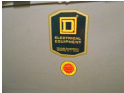
Basement electrical main
