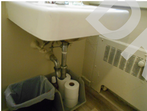
Building A, Unit 9, 1br/1ba - Bathroom sink, no scald abrasion protection
