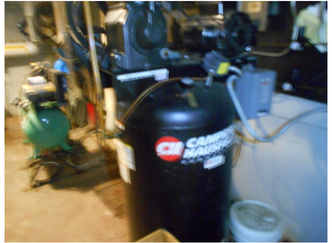
58. Basement mechanical room, pumps
