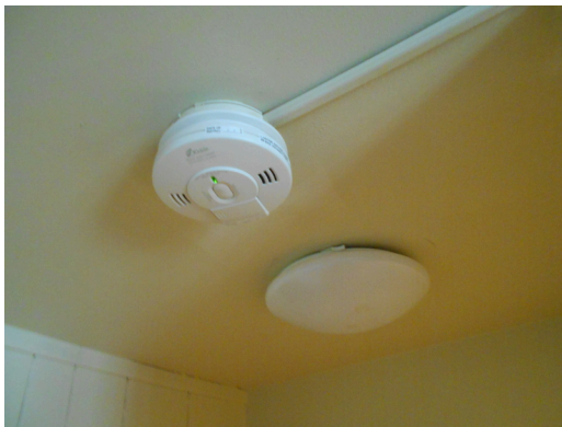
Building B, Unit 23, 1br/1ba - Living area smoke detector
