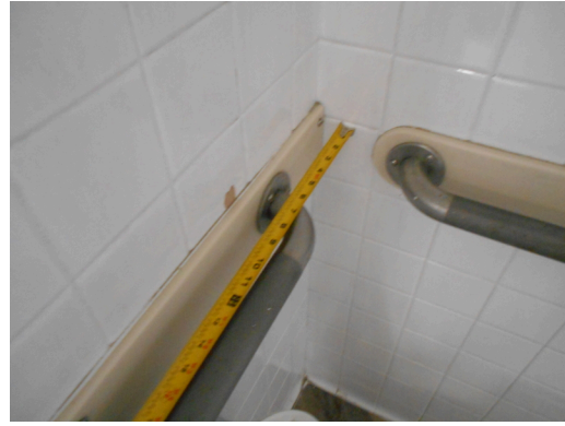
Men's public restroom, rear grab bar
