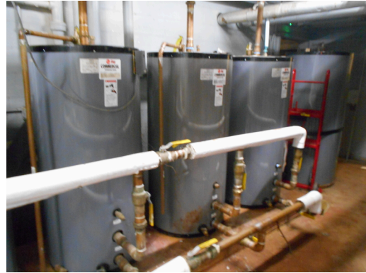
Basement mechanical room, hot water storage tanks
