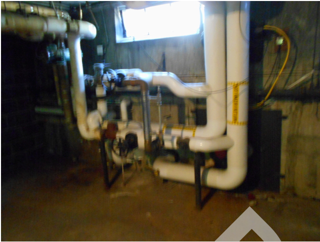
61. Building A water main
