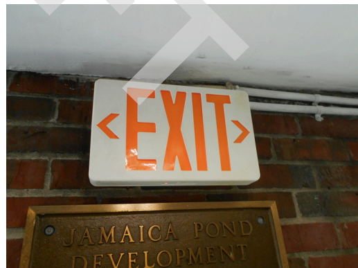
Emergency exit sign
