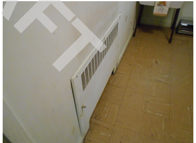
28. Building B, Unit 27, 2br/1ba - Living area radiator
