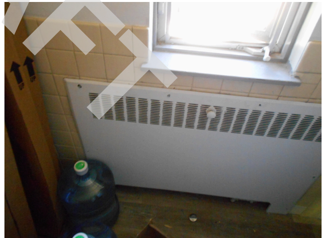
44. Community building steam radiator
