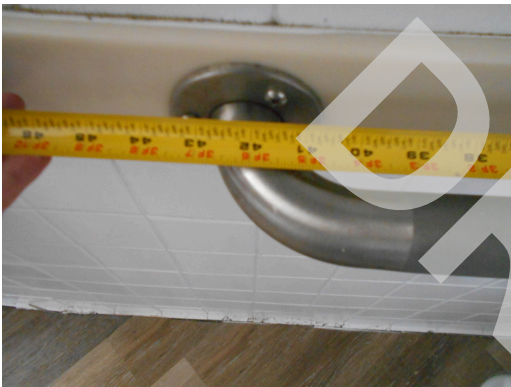
Men's public restroom, rear grab bar, 42"
