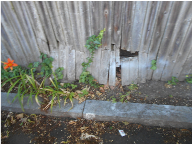
11. Parking lot wood fencing, damaged (Non-Critical Repair)
