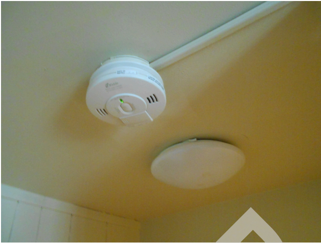
41. Building B, Unit 23, 1br/1ba - Living area smoke detector
