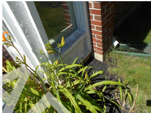
Community building window, paint chipping (Non-Critical Repair)
