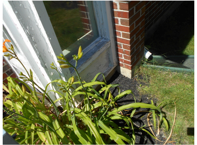
18. Community building window, paint chipping (Non-Critical Repair)
