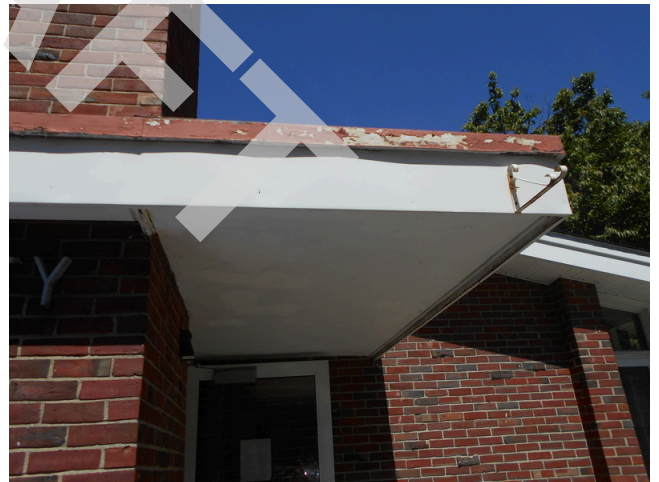
16. Community building, paint chipping (Non-Critical Repair)
