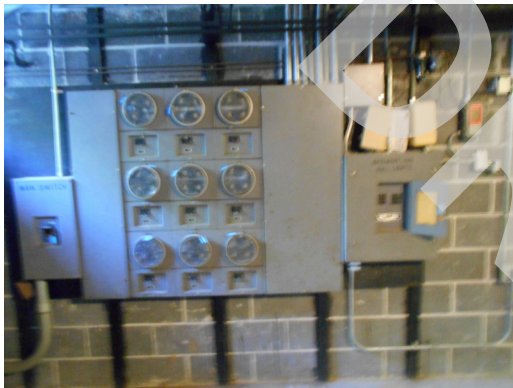
Building A electrical meters
