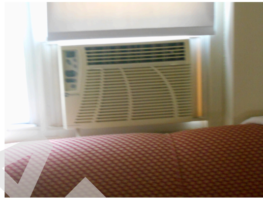
Building B, Unit 23, 1br/1ba - Window A/C unit
