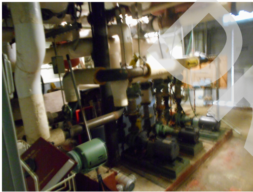
Basement mechanical room, circulation pumps
