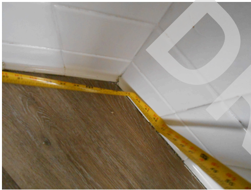
Men's public restroom, not enough clear floor space (Critical Repair)
