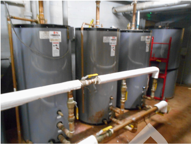
49. Basement mechanical room, hot water storage tanks
