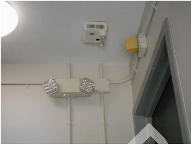
105. Typical stairwell fire alarm and emergency light
