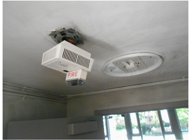
26. Community building fire alarm
