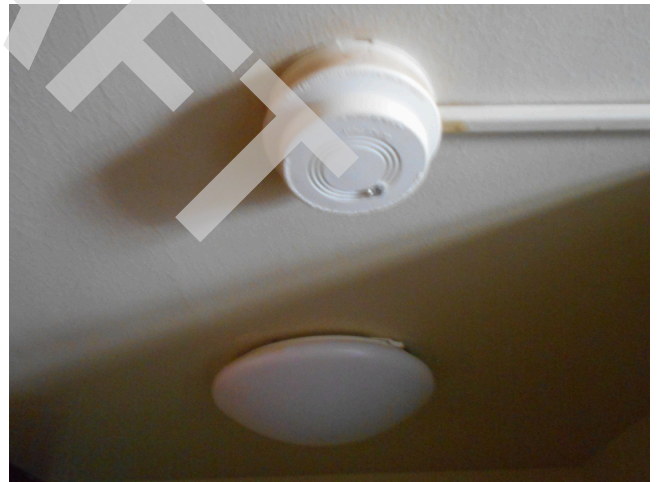
20. Building A, Unit 7, 1br/1ba - Living area area smoke detector
