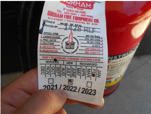
107. Fire extinguisher, inspected February 2022
