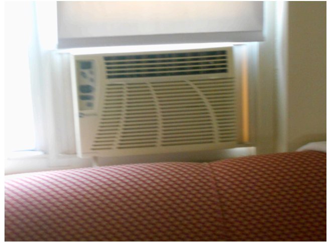
46. Building B, Unit 23, 1br/1ba - Window A/C unit
