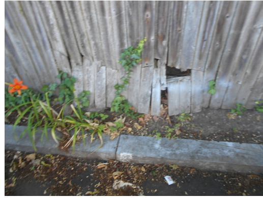
Parking lot wood fencing, damaged (Non-Critical Repair)
