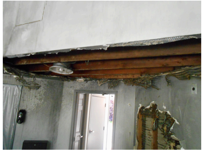
38. Community building main room, damaged by fire (Non-Critical Repair)
