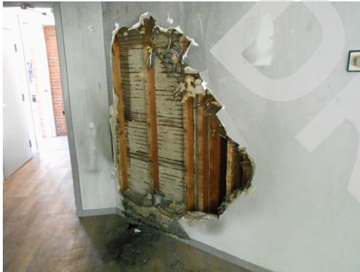
Community building main room, damaged by fire (Non-Critical Repair)
