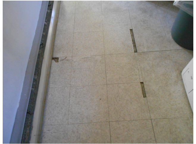
42. Community building laundry room, chipped vinyl tile floor (Non-Critical Repair)
