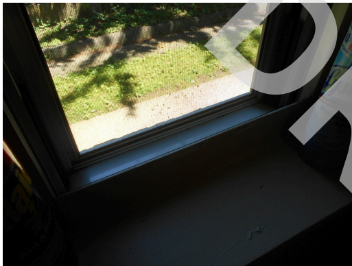
Building A, Unit 9, 1br/1ba - Typical window
