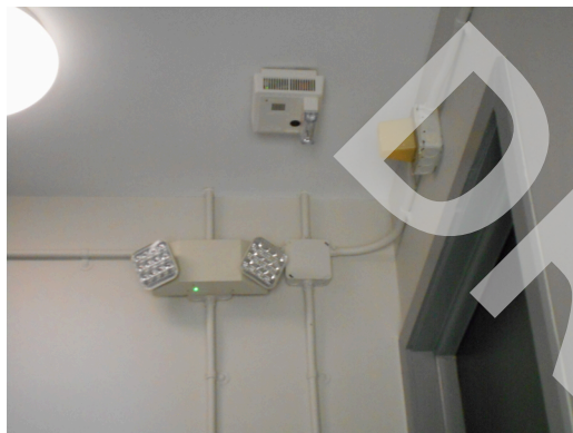
Typical stairwell fire alarm and emergency light
