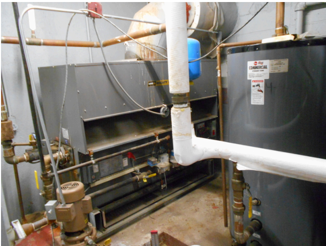
47. Basement mechanical room, water heater
