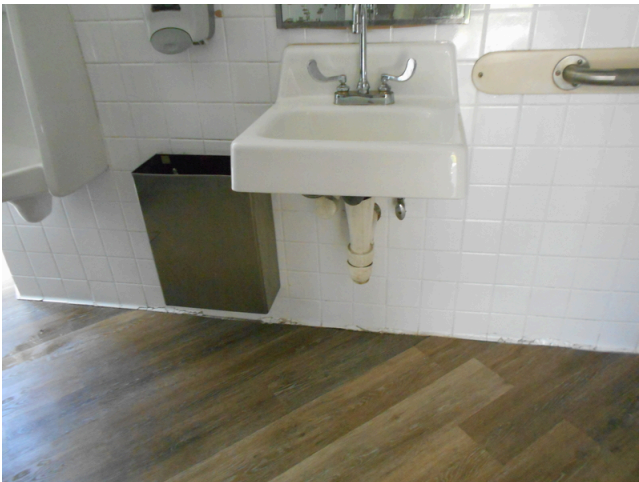
31. Men's public restroom, no scald abrasion protection (Critical Repair)
