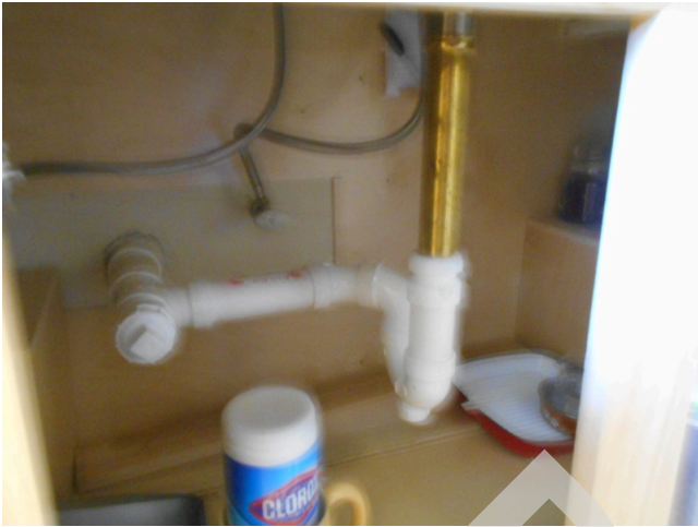
5. Building A, Unit 9, 1br/1ba - Kitchen sink piping
