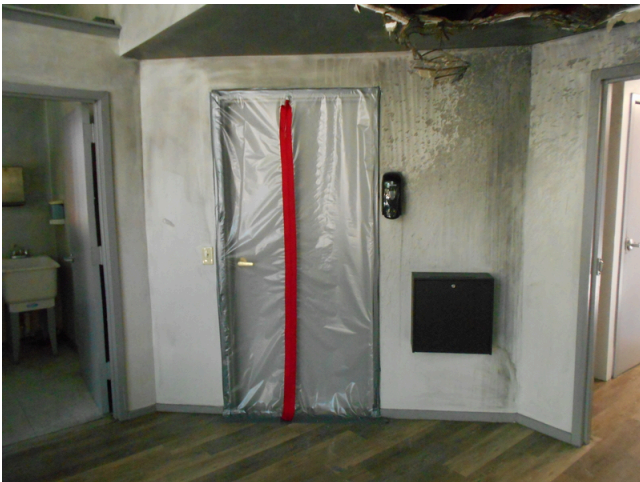
39. Community building main room, damaged by fire (Non-Critical Repair)
