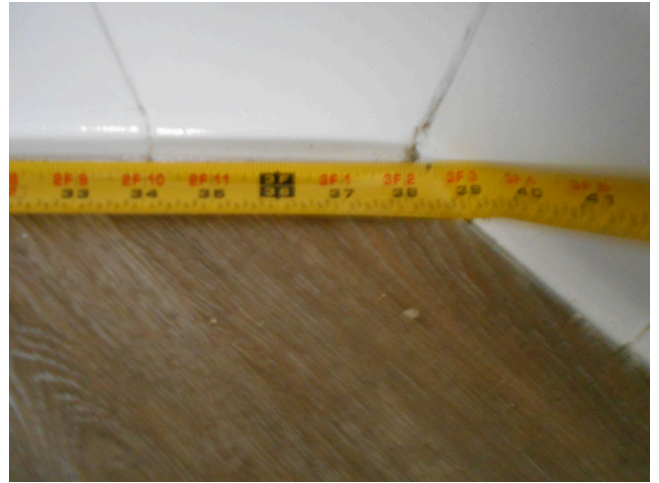
30. Men's public restroom, not enough clear floor space (Critical Repair)
