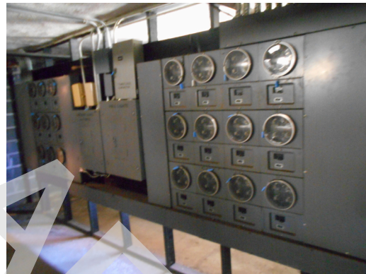
Building D basement electrical meters
