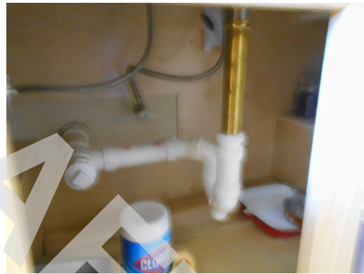
Building A, Unit 9, 1br/1ba - Kitchen sink piping
