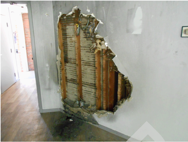
37. Community building main room, damaged by fire (Non-Critical Repair)
