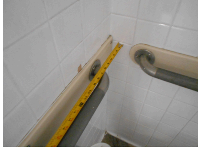
34. Men's public restroom, rear grab bar
