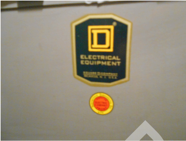
53. Basement electrical main
