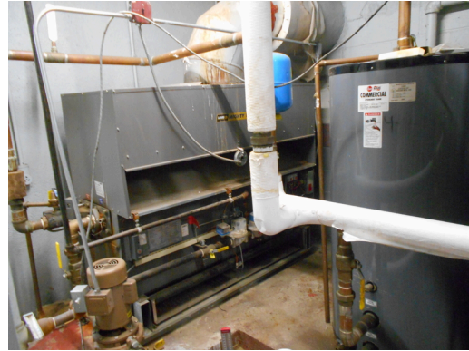
Basement mechanical room, water heater
