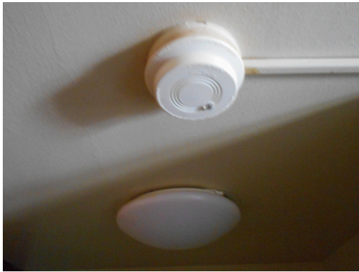
Building A, Unit 7, 1br/1ba - Living area area smoke detector
