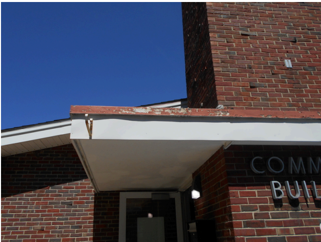
15. Community building, paint chipping (Non-Critical Repair)
