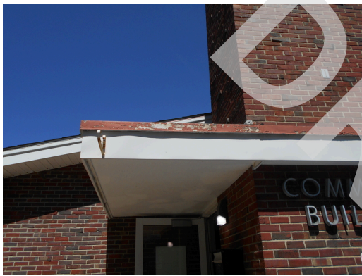
Community building, paint chipping (Non-Critical Repair)
