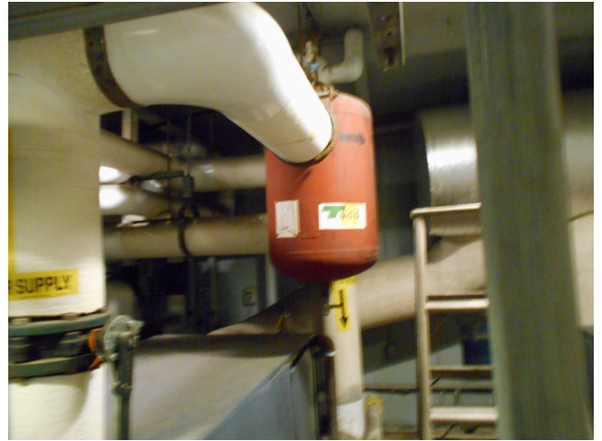
54. Basement mechanical room, expansion tank
