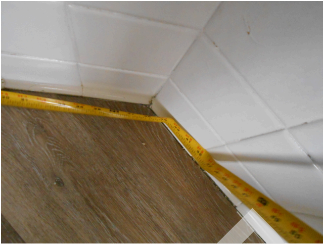
29. Men's public restroom, not enough clear floor space (Critical Repair)
