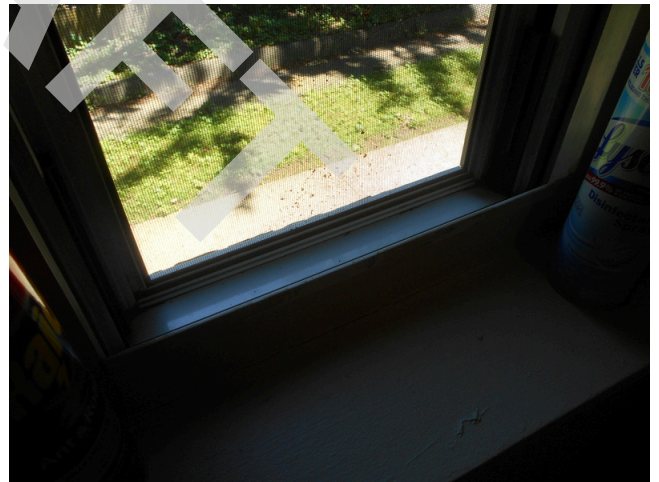
8. Building A, Unit 9, 1br/1ba - Typical window
