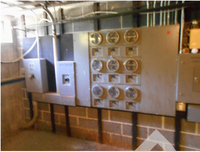
65. Building B basement electric meters
