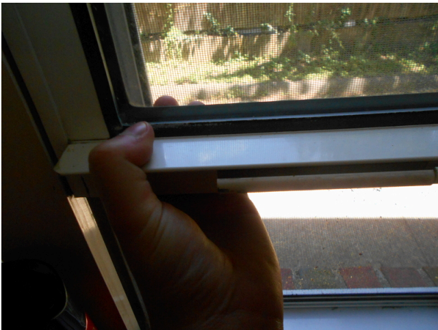
7. Building A, Unit 9, 1br/1ba - Typical window
