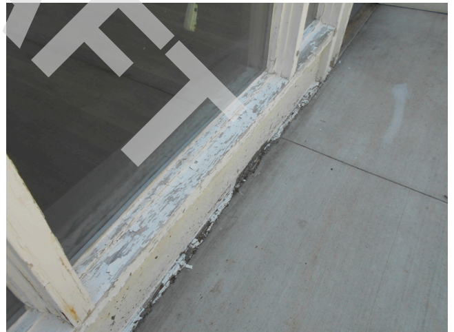
20. Community building rear façade, paint chipping (Non-Critical Repair)
