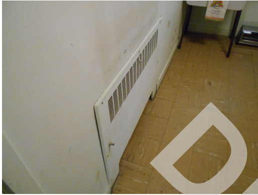
Building B, Unit 27, 2br/1ba - Living area radiator
