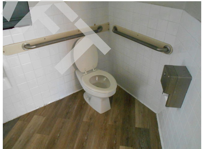
28. Men's public restroom, not enough clear floor space (Critical Repair)
