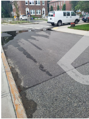
Property parking lot ingress/egress (Non-Critical Repair)
