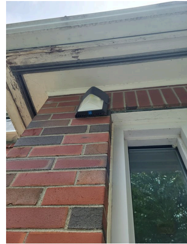
62. Apartment building 342-356 wood soffit damage
