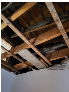
Common area restroom hole in ceiling (Non-Critical Repair)
