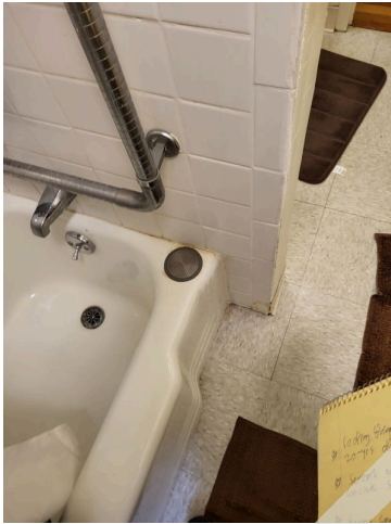
49. Apartment 354-21 bathroom bathtub tile damage (Non-Critical Repair)
