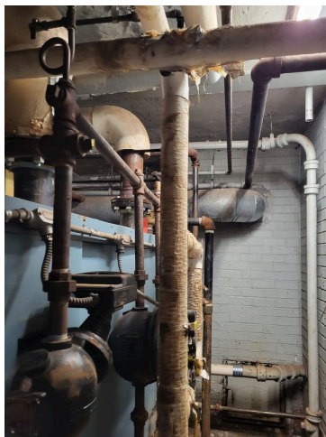
99. Cast iron pipes
