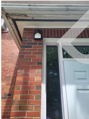
Apartment building 342-356 ingress/egress light fixture
