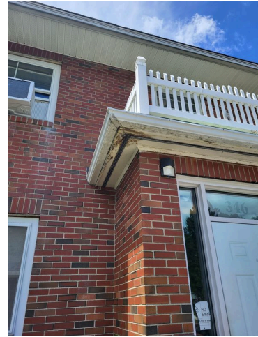
78. Apartment building 342-356 wood soffit damage (Non-Critical Repair)
