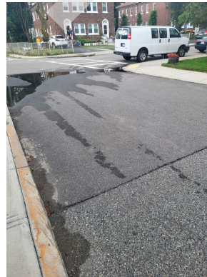
Property parking lot ingress/egress (Non-Critical Repair)
