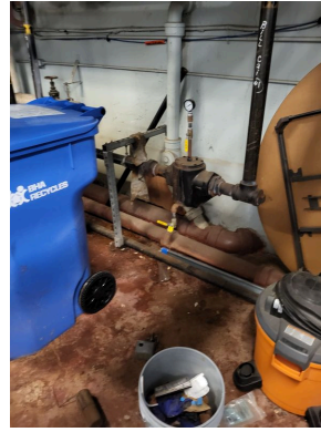
Maintenance area circulation pump
