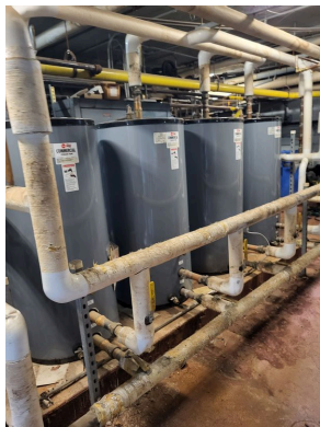
Hot water storage tanks (115 gallon each)
