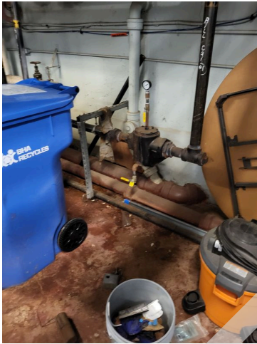
109. Maintenance area circulation pump
