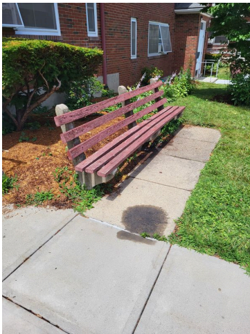
79. Exterior common area bench (Non-Critical Repair)
