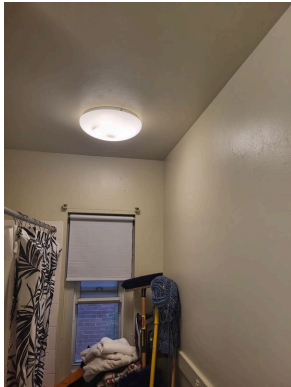
Apartment 364-36 bathroom light fixture and window
