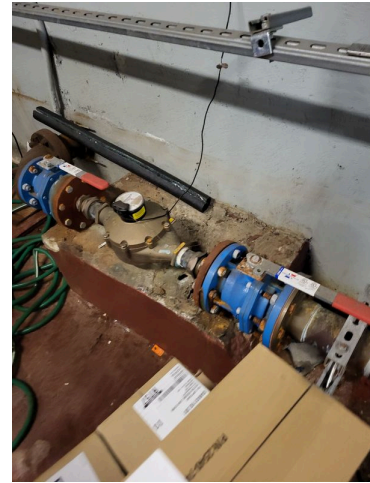
110. Maintenance area circulation pump
