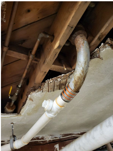
119. Basement ceiling damage (Non-Critical Repair)
