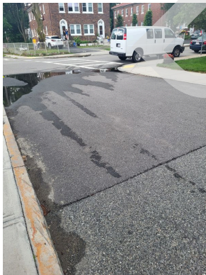
Property parking lot ingress/egress (Non-Critical Repair)
