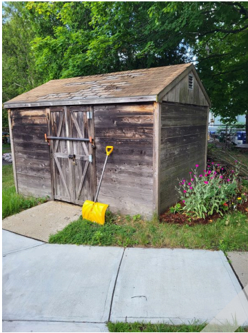
137. Property concrete sidewalk replacement connecting to older concrete sidewalk trip hazard (Critical Repair)
