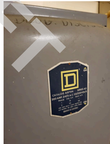
128. Apartment building 342 circuit breaker box
