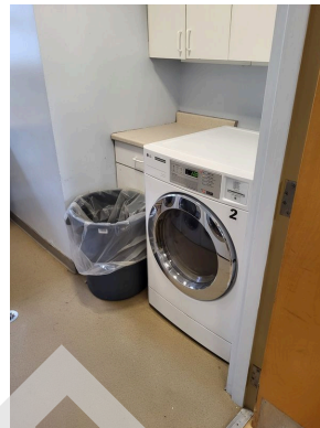
Common area laundry room front load dryer
