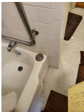
Apartment 354-21 bathroom bathtub tile damage (Non-Critical Repair)
