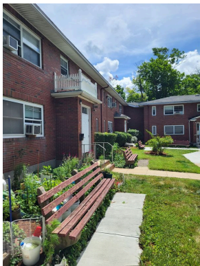
Exterior common area benches (Non-Critical Repair)
