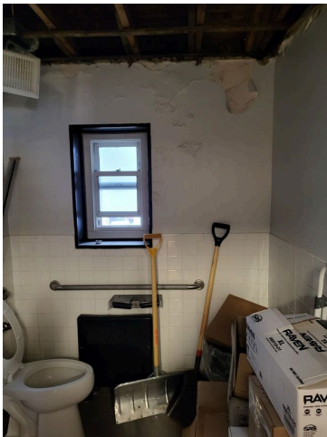
47. Common area restroom ceiling damage (Non-Critical Repair)
