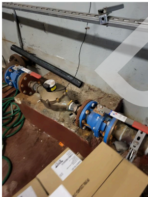
Maintenance area circulation pump
