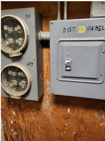
143. Basement apartment building distribution panel
