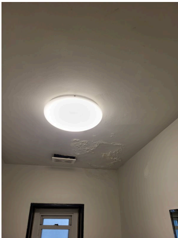
67. Apartment building 342-356 common area light fixture and ceiling damage (Non-Critical Repair)
