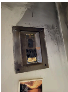
Apartment 370-46 circuit breakers (Non-Critical Repair)
