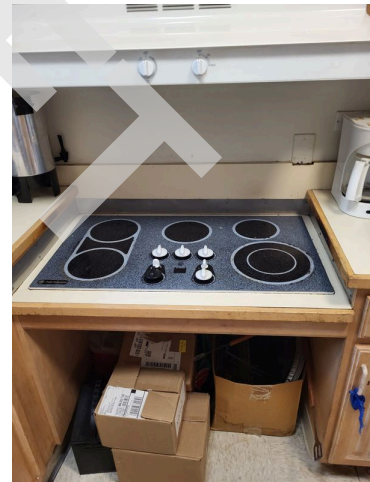
20. Common area kitchen range burners
