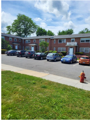
Property parking lot (Non-Critical Repair)
