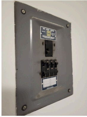
Apartment 374-54 circuit breakers
