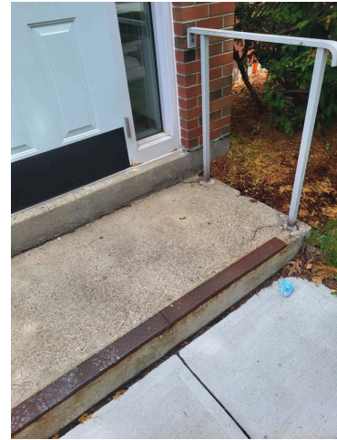
66. Apartment building 342-356 cracked concrete by stair railing (Non-Critical Repair)
