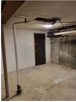
Basement damaged ceiling (Non-Critical Repair)
