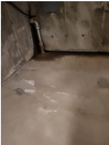
123. Basement pipe leak (Non-Critical Repair)
