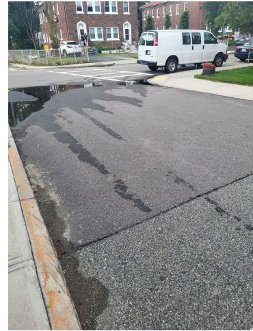
86. Property parking lot ingress/egress (Non-Critical Repair)
