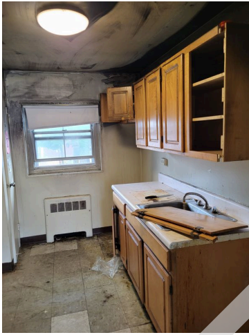
69. Apartment 370-46 kitchen fire and smoke damage (Non-Critical Repair)
