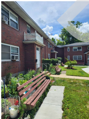
Exterior common area benches (Non-Critical Repair)
