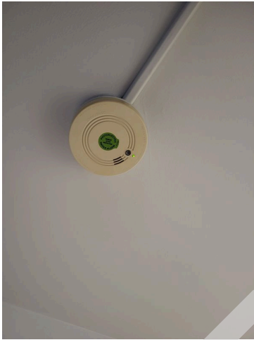
105. Apartment 374-54 smoke detector
