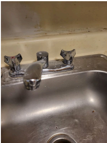
63. Apartment 356-25 kitchen sink and faucet
