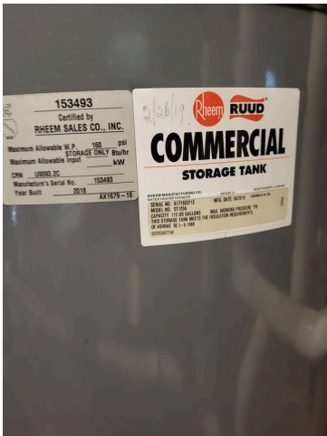
91. Hot water storage tank
