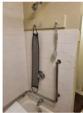
Apartment 354-21 bathroom bathtub hardware
