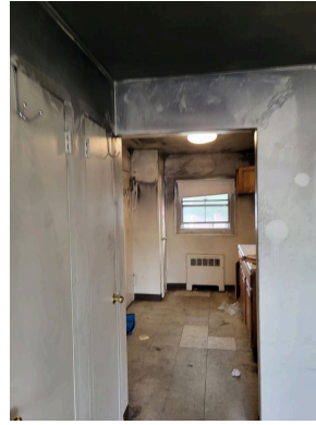
Apartment 370-46 fire and smoke damage (Non-Critical Repair)
