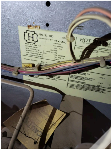
93. Hot water boiler
