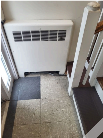
125. Apartment 342-1 breezeway radiator
