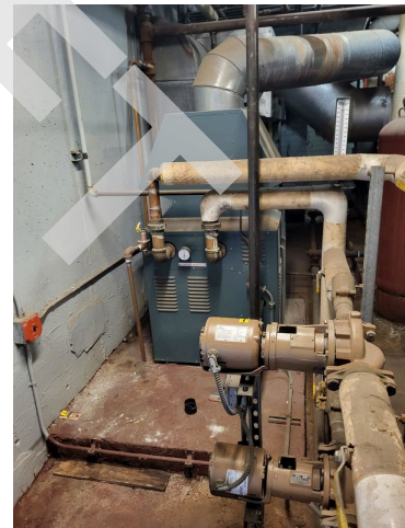
92. Hot water boiler (726,000 btu)
