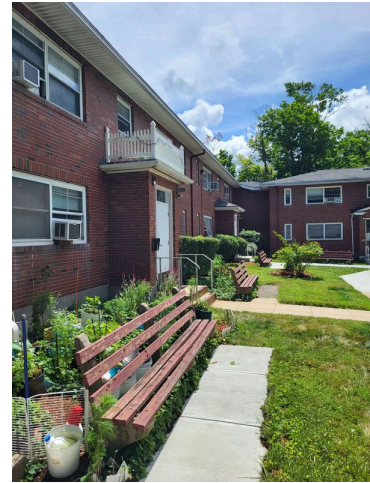
82. Exterior common area benches (Non-Critical Repair)
