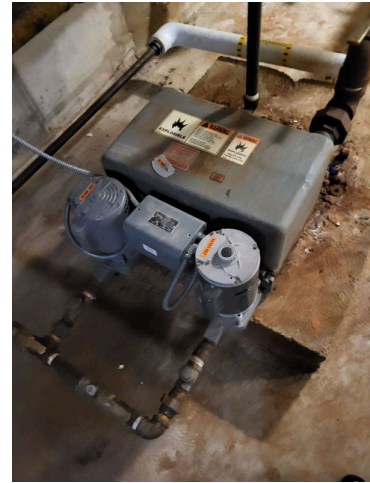
146. Basement apartment building boiler system condensate pump
