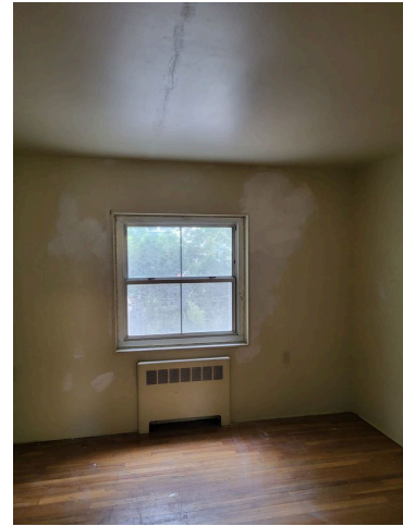
58. Apartment 356-25 bedroom missing smoke detector (Critical Repair)
