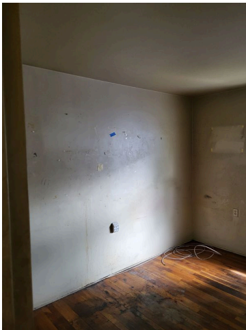
75. Apartment 370-46 smoke damage (Non-Critical Repair) Missing smoke detector (Critical Repair)
