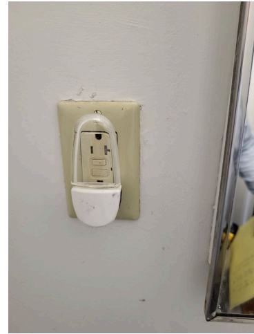
38. Apartment 352-19 bathroom GFCI
