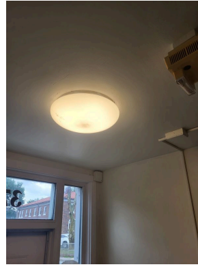
Apartment building 358-374 common area light fixture
