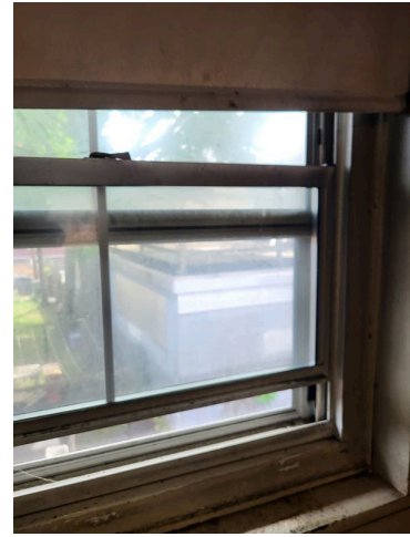
70. Apartment 370-46 kitchen window and frame (Non-Critical Repair)
