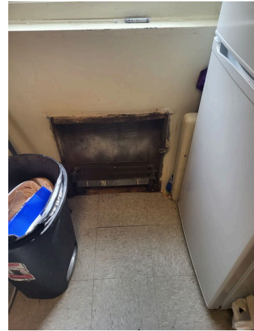
78. Apartment 364-36 kitchen radiator missing cover (Non-Critical Repair)
