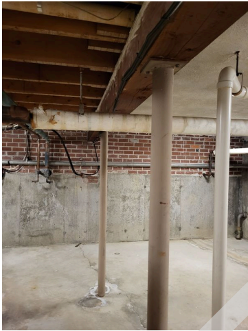
121. Basement ceiling damage (Non-Critical Repair)
