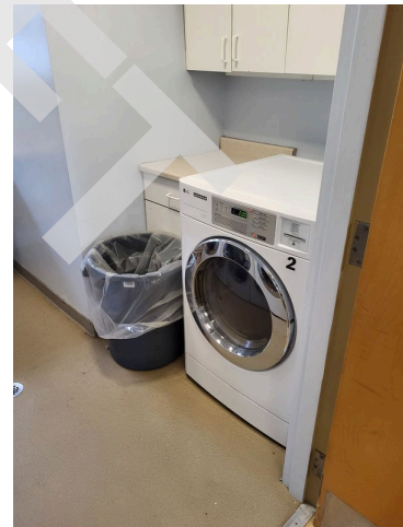
12. Common area laundry room front load dryer
