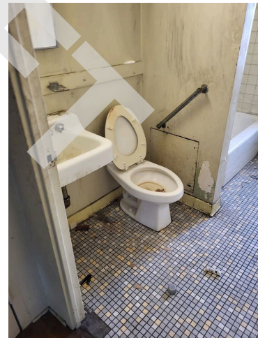
72. Apartment 370-46 bathroom toilet, grab bar, sink and floor (Non-Critical Repair)
