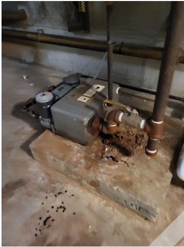
145. Basement apartment building boiler system condensate pump
