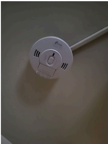
83. Apartment 364-36 hallway smoke detector
