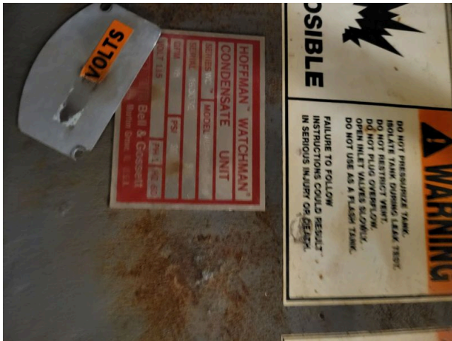
147. Basement apartment building boiler system condensate pump
