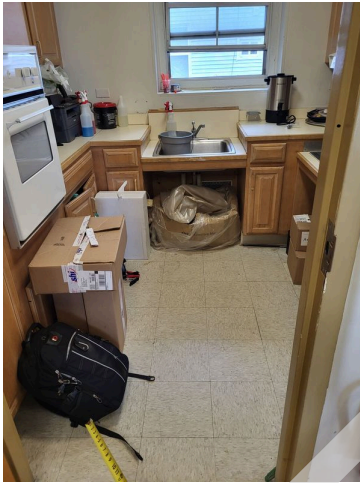
25. Common area kitchen are flooring (Non-Critical Repair)
