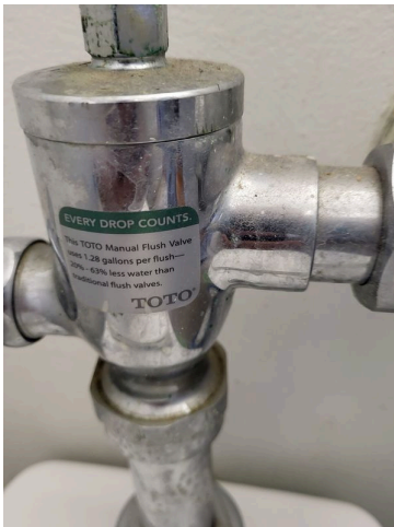
35. Apartment 352-19 efficiency control flush valve
