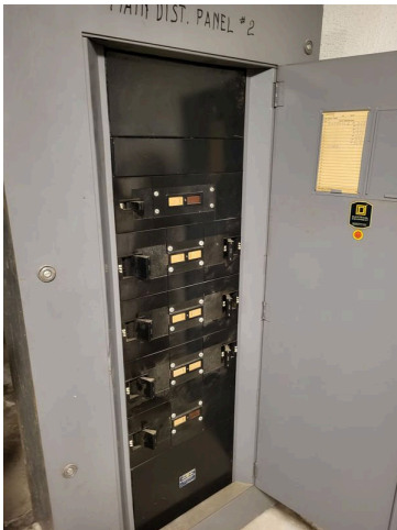
151. Apartment building main distribution panel two (2)
