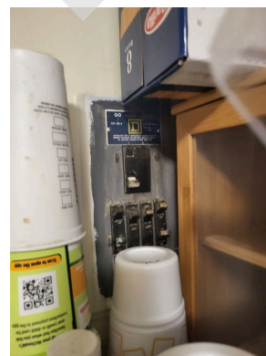
Apartment 364-36 circuit breakers
