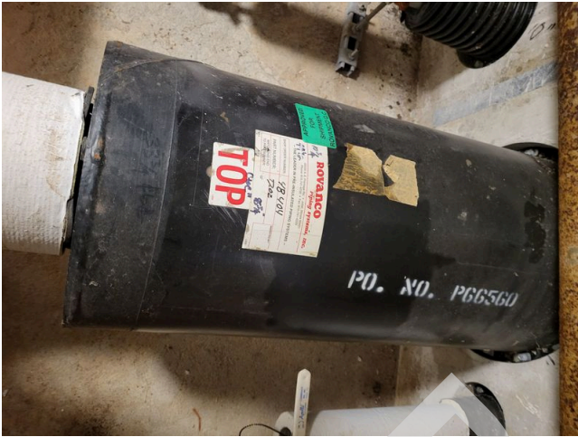
149. Basement steam supply pump
