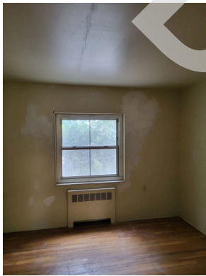
Apartment 356-25 bedroom missing smoke detector (Critical Repair)
