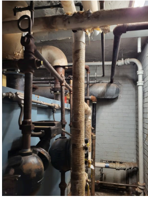
Cast iron pipes
