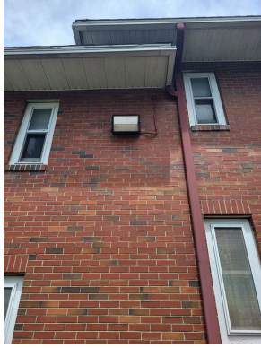
Apartment building 342-356 wall mounted high intensity light fixture
