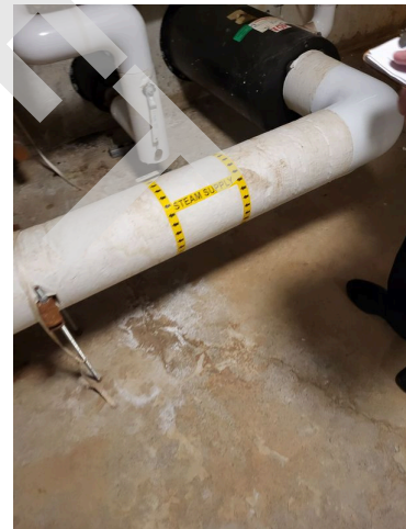
148. Basement steam supply pipe
