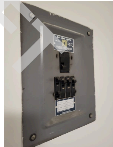
104. Apartment 374-54 circuit breakers
