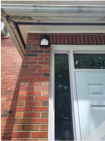
61. Apartment building 342-356 ingress/egress light fixture
