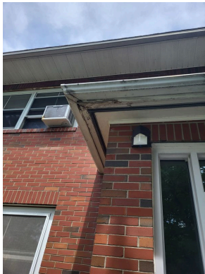
Apartment building 342-356 wood soffit damage (Non-Critical Repair)
