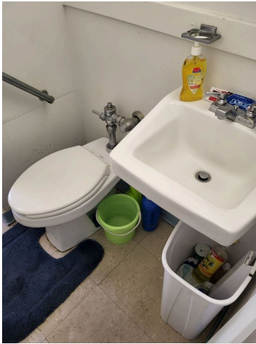
33. Apartment 352-19 bathroom toilet, sink and faucet
