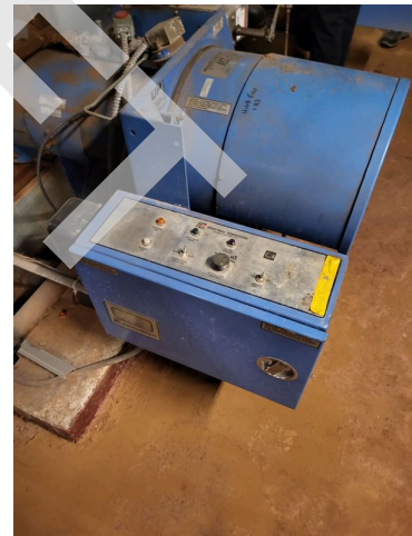
96. Boiler number one (1)
