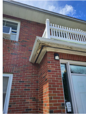
Apartment building 342-356 wood soffit damage (Non-Critical Repair)
