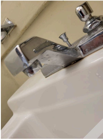
17. Apartment 346-10 bathroom sink faucet
