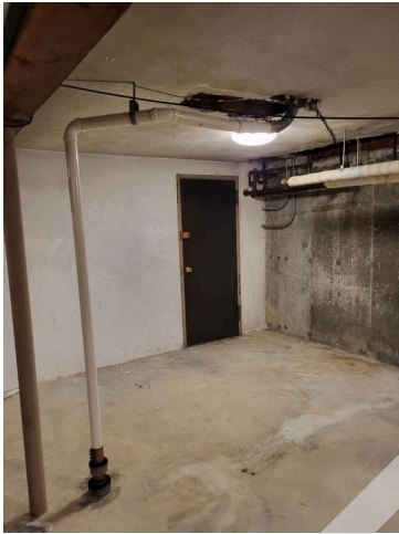
113. Basement damaged ceiling (Non-Critical Repair)
