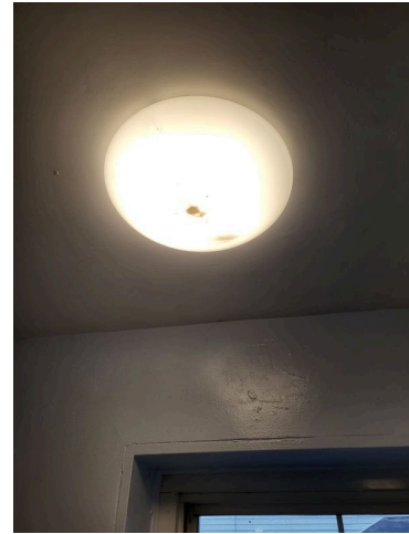
14. Common area laundry room light fixture
