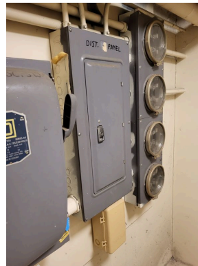
Apartment building 342 distribution panel
