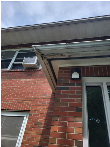
63. Apartment building 342-356 wood soffit damage (Non-Critical Repair)
