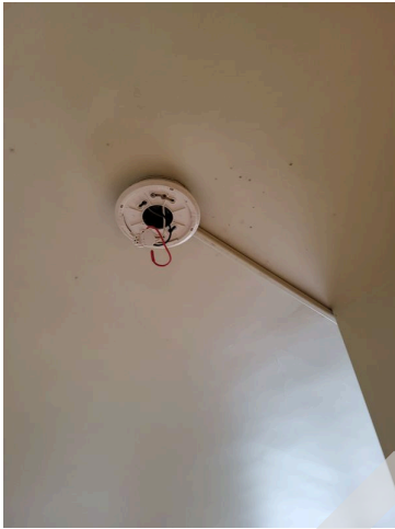
61. Apartment 356-25 missing smoke detector (Critical Repair)
