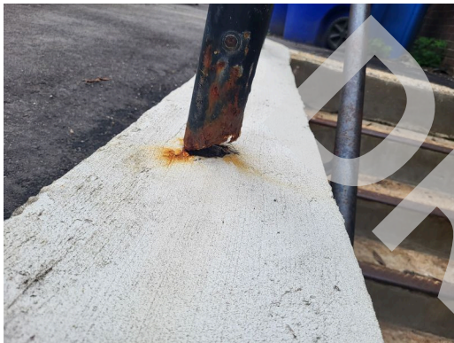
Basement ingress/egress railing rusted (Non-Critical Repair)
