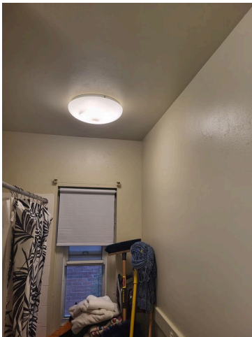
91. Apartment 364-36 bathroom light fixture and window
