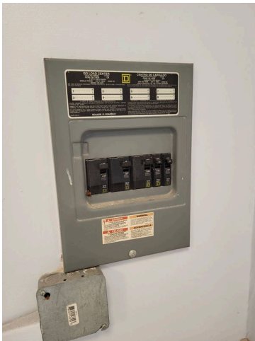
15. Common area circuit breaker box
