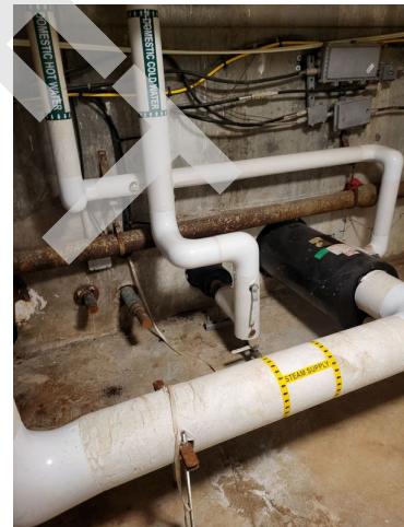
144. Basement apartment building pipes
