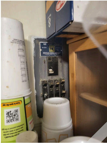
81. Apartment 364-36 circuit breakers
