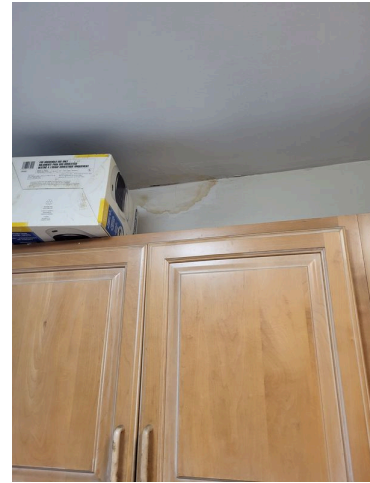
22. Common area kitchen ceiling damage (Non-Critical Repair)
