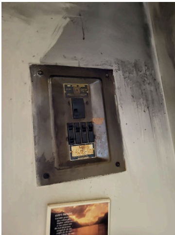
71. Apartment 370-46 circuit breakers (Non-Critical Repair)
