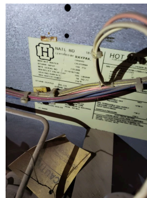
Hot water boiler
