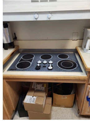
Common area kitchen range burners
