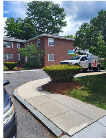
166. Property sidewalk trip hazard (Critical Repair)
