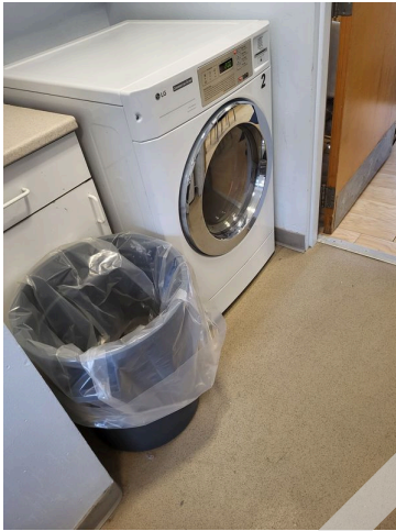
13. Common area laundry room front load dryer
