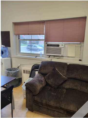
45. Common area room window mounted air conditioner
