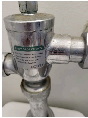
Apartment 352-19 efficiency control flush valve
