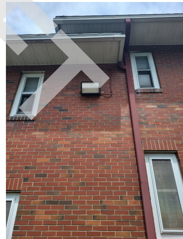
64. Apartment building 342-356 wall mounted high intensity light fixture
