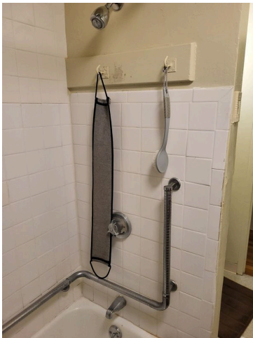
47. Apartment 354-21 bathroom bathtub hardware
