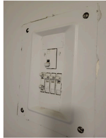
30. Apartment 352-19 circuit breakers
