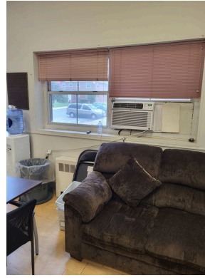
Common area room window mounted air conditioner
