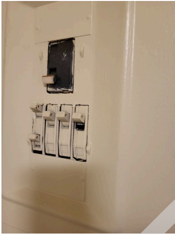
41. Apartment 354-21 circuit breakers
