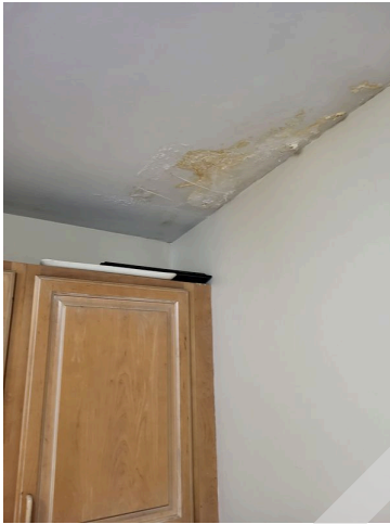
21. Common area kitchen ceiling damage (Non-Critical Repair)
