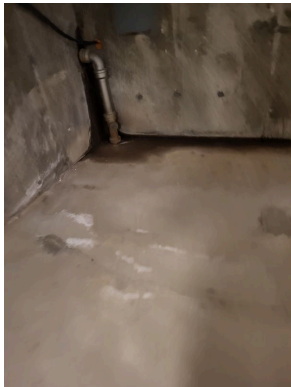
Basement pipe leak (Non-Critical Repair)
