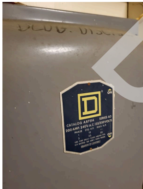
Apartment building 342 circuit breaker box
