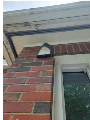
Apartment building 342-356 wood soffit damage
