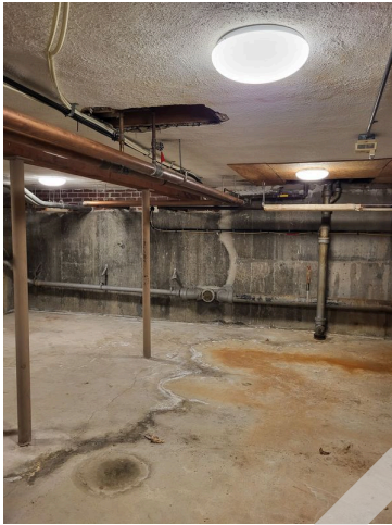
153. Basement light fixtures
