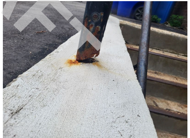
72. Basement ingress/egress railing rusted (Non-Critical Repair)
