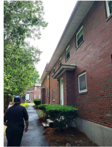
130. Apartment building wood soffit and trim damage (Non-Critical Repair)
