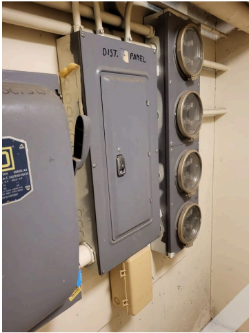
129. Apartment building 342 distribution panel
