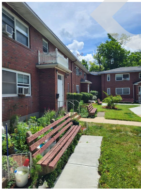
Exterior common area benches (Non-Critical Repair)
