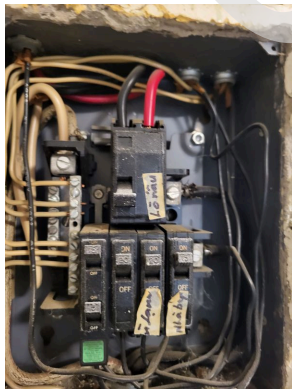
Apartment 356-25 circuit breakers and wiring
