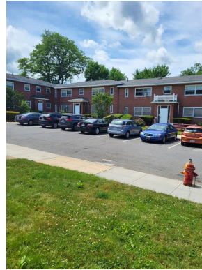
Property parking lot (Non-Critical Repair)
