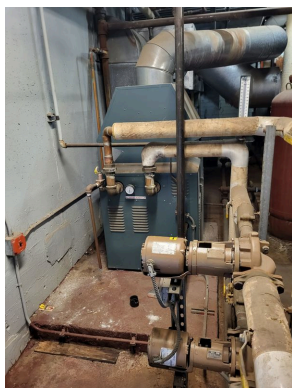
Hot water boiler (726,000 btu)
