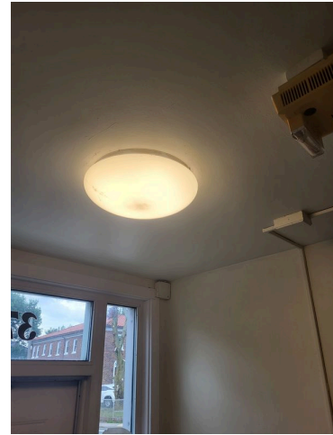
102. Apartment building 358-374 common area light fixture
