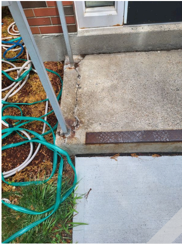
65. Apartment building 342-356 cracked concrete by stair railing (Non-Critical Repair)
