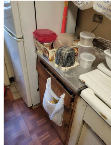
10. Apartment 346-10 countertop and cabinets (Non-Critical Repair)
