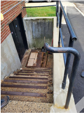
73. Basement ingress/egress railing damaged (Non-Critical Repair)
