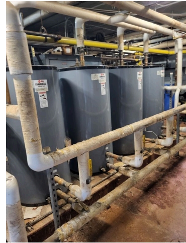
90. Hot water storage tanks (115 gallon each)
