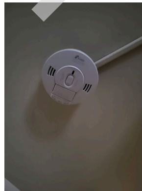
Apartment 364-36 hallway smoke detector
