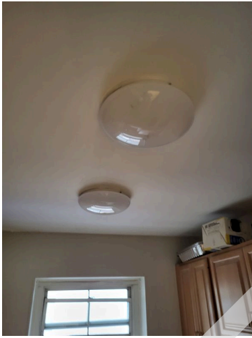
17. Common area kitchen light fixtures
