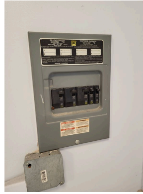
Common area circuit breaker box
