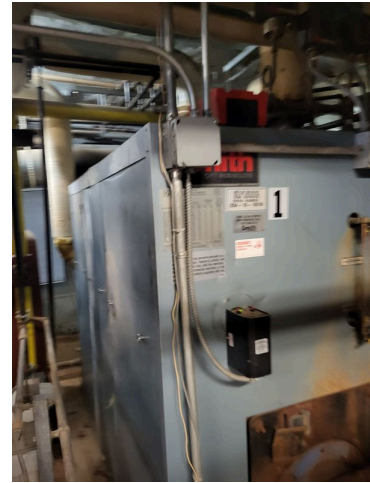
94. Boiler number one (1)
