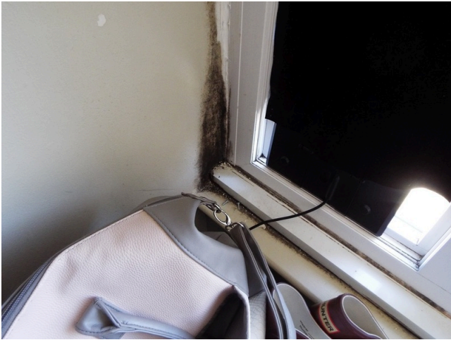
122. 1-bed-1-bath - unit 32 - building 105-109, mildew around frames
