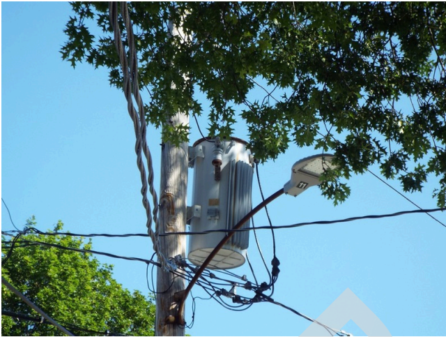
17. Pole mounted transformer
