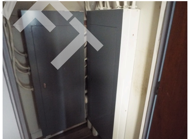
84. Electrical room - building 105-109
