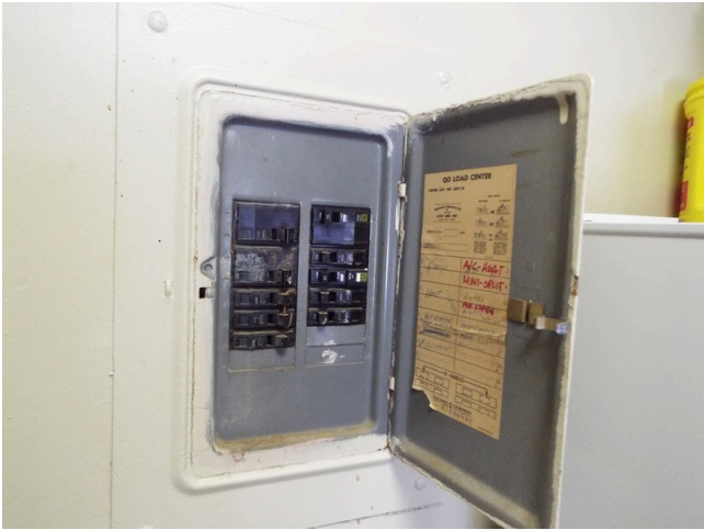
114. Typical unit electrical panel
