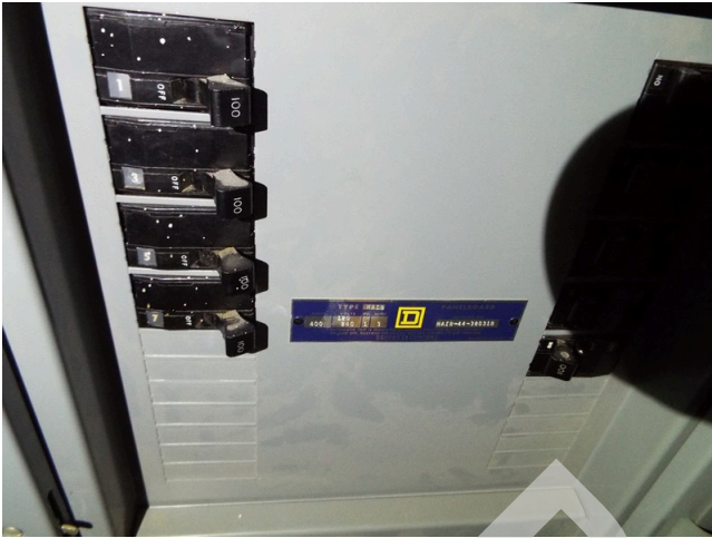
41. Building electrical panel - building 93-95
