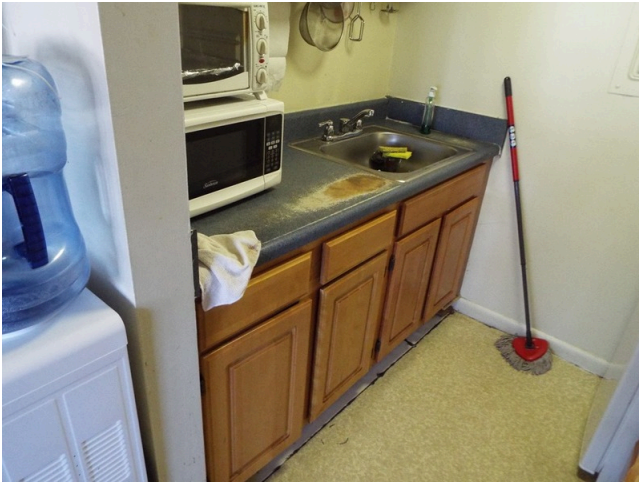
111. 1-bed-1-bath - unit 32 - building 105-109 - countertop condition (Non-Critical Repair)
