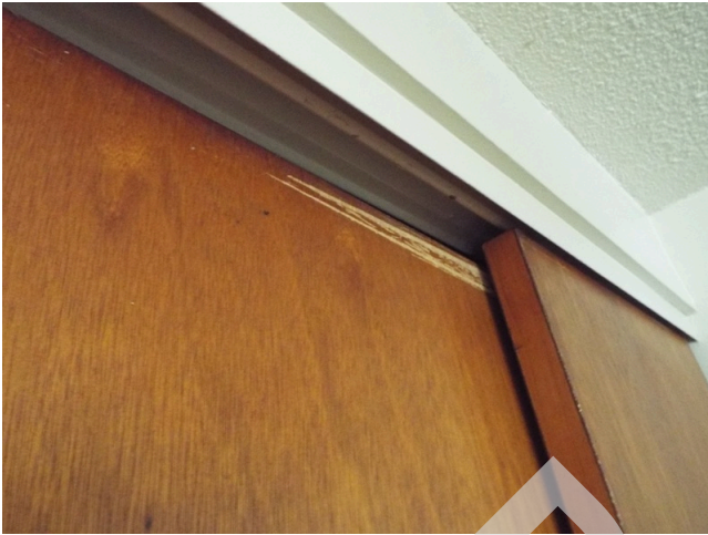
93. 0-bed-1-bath - unit 25 - building 105-109 - closet door hanger detached (Non-Critical Repair)
