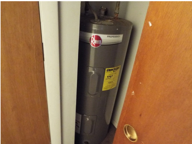
15. 0-bed-1-bath - unit 13 - building 93-95 - water heater
