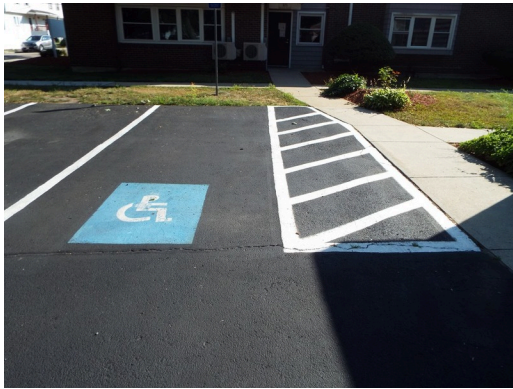
Accessible parking lacks van space and sign (Critical Repair)
