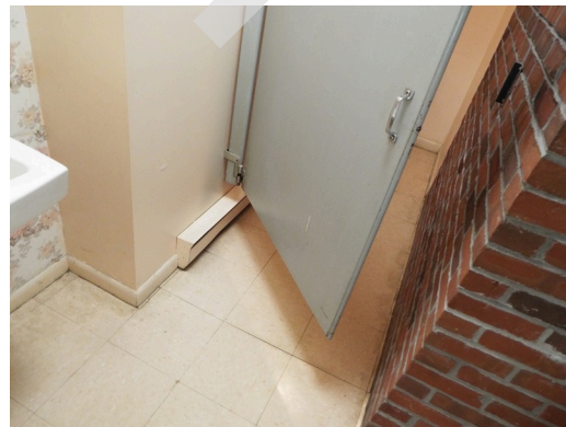
Community building - mens room lacks 60 inch turning clearance (Critical Repair)
