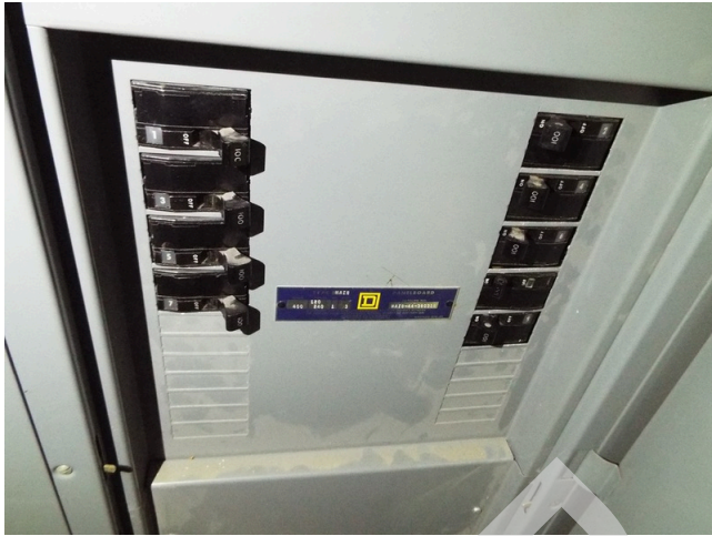
85. Electrical room - building 105-109
