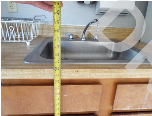
Community building - sink exceeds 34 inch maximum height (Critical Repair)
