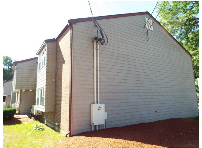
18. Building electrical service and meter
