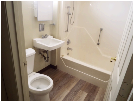
0-bed-1-bath - unit 41 - building 110-112- bathroom fixtures
