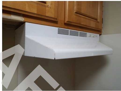
0-bed-1-bath - unit 41 - building 110-112 - range hood
