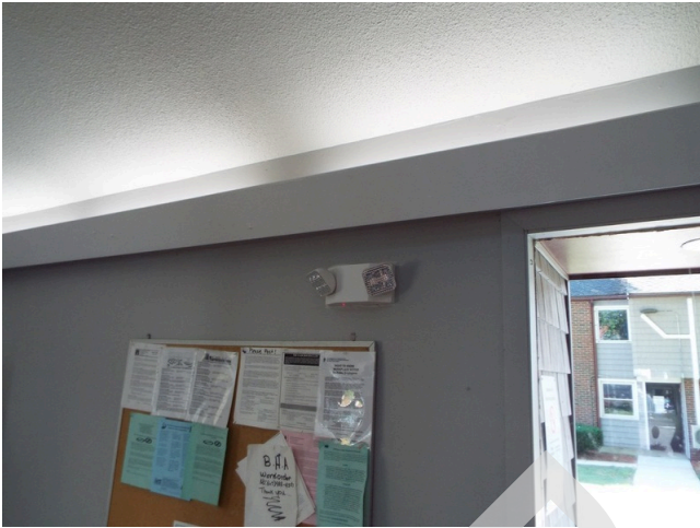
45. Community building - emergency lights
