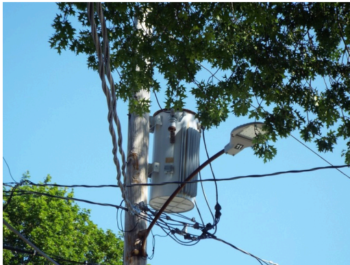
Pole mounted transformer
