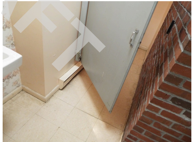
60. Community building - mens room lacks 60 inch turning clearance (Critical Repair)
