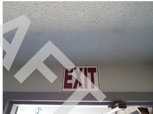
Building hallway exit sign
