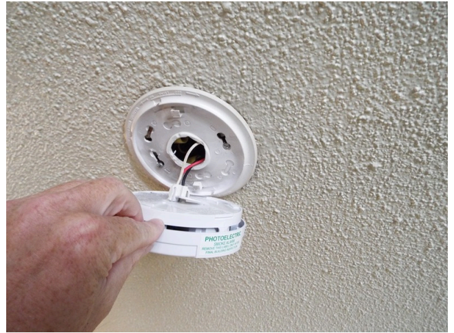
74. Typical unit hardwired smoke detector
