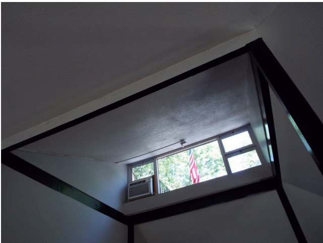
39. Community building - window mounted HVAC unit
