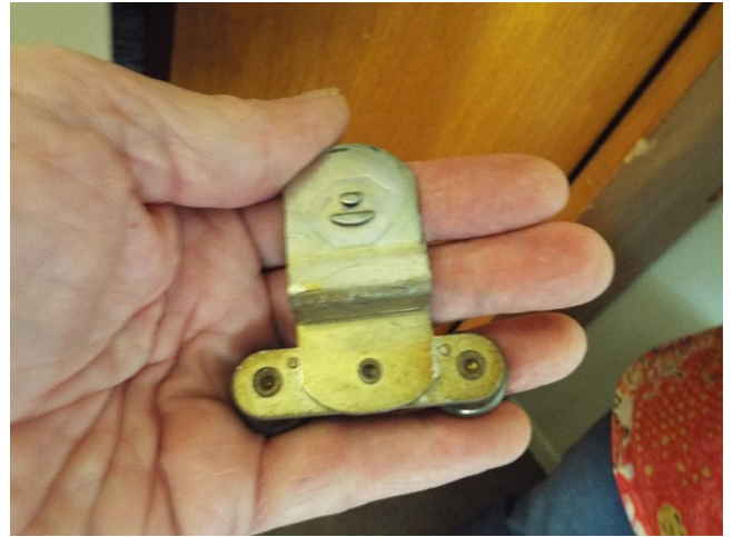
94. 0-bed-1-bath - unit 25 - building 105-109 - closet door hanger detached (Non-Critical Repair)
