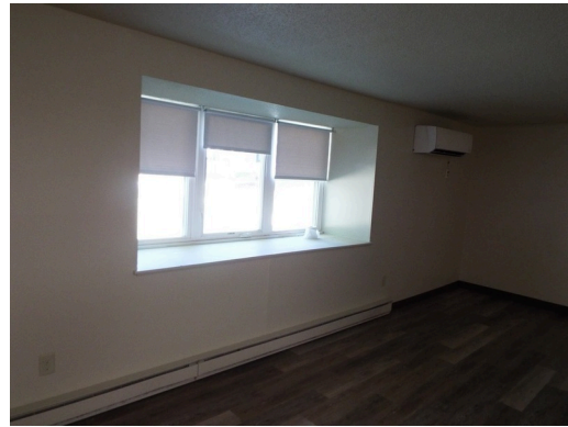
Unit electric baseboard (emergency use)
