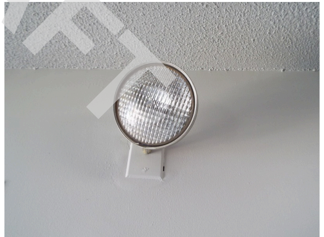
44. Building hallway emergency light
