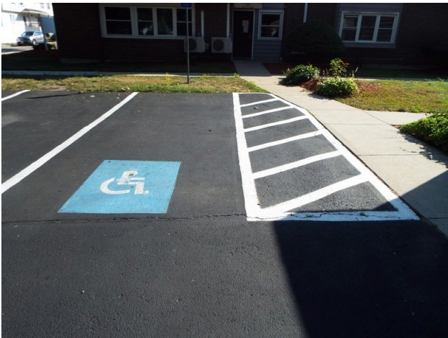
55. Accessible parking lacks van space and sign (Critical Repair)
