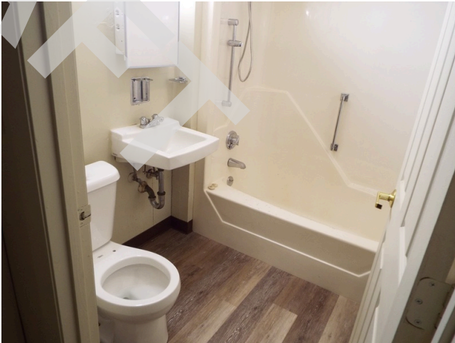
168. 0-bed-1-bath - unit 41 - building 110-112- bathroom fixtures
