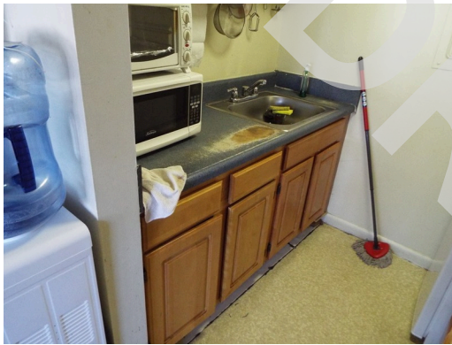
1-bed-1-bath - unit 32 - building 105-109 - countertop condition (Non-Critical Repair)
