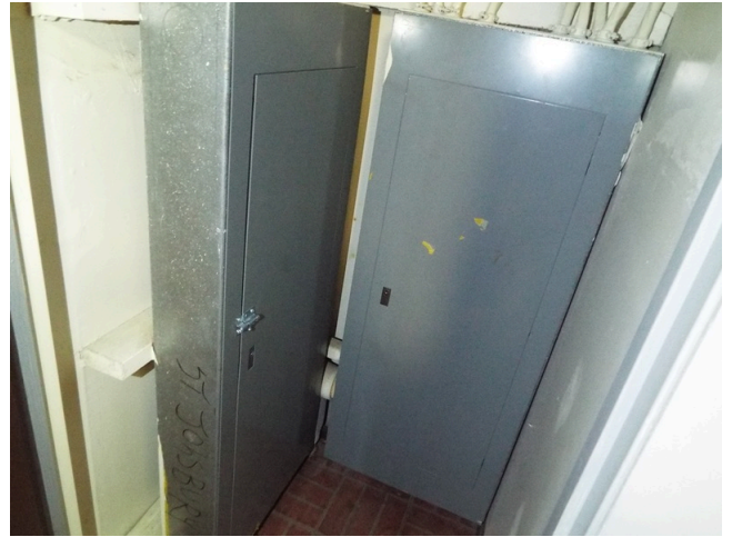
66. Electrical room - building 93-95
