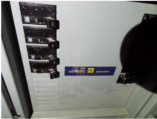
Building electrical panel - building 93-95
