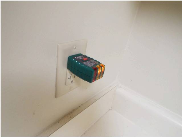
185. Kitchen GFCI operates correctly
