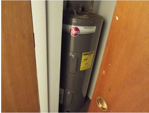
0-bed-1-bath - unit 13 - building 93-95 - water heater
