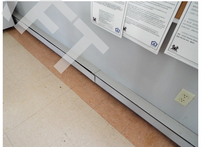
40. Community building - electric baseboard
