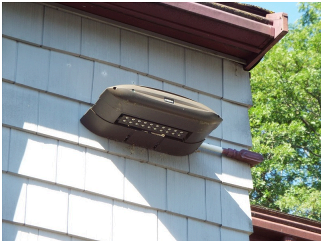
11. Building mounted lighting
