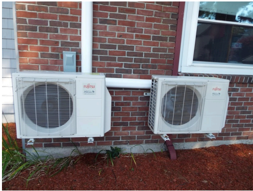
Typical mini-split heat pumps
