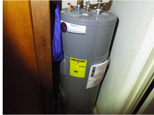
1-bed-1-bath - unit 12 - building 93-95 - water heater
