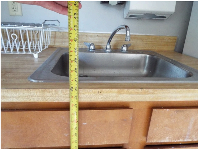
63. Community building - sink exceeds 34 inch maximum height (Critical Repair)
