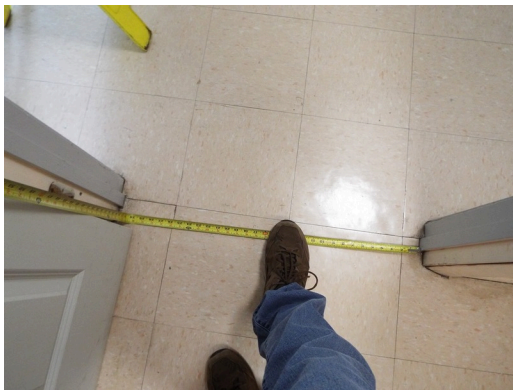
Community building - mens room door lacks minum 32 inch clearance (Critical Repair)
