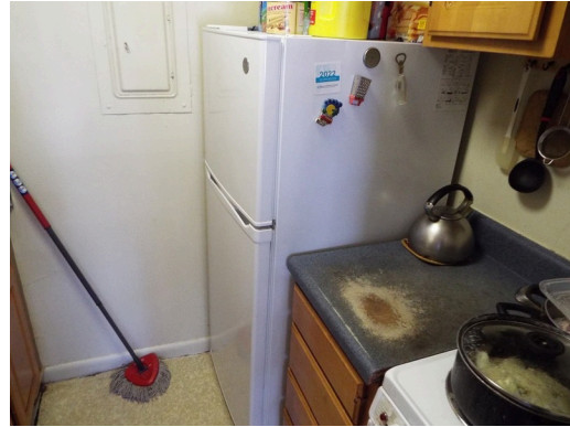
1-bed-1-bath - unit 32 - building 105-109 - countertop condition (Non-Critical Repair)
