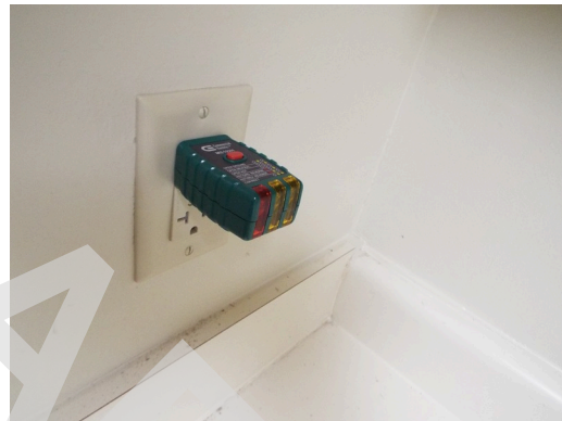
Kitchen GFCI operates correctly
