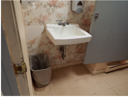
Community building - mens room sink lacks pipe protection (Critical Repair)
