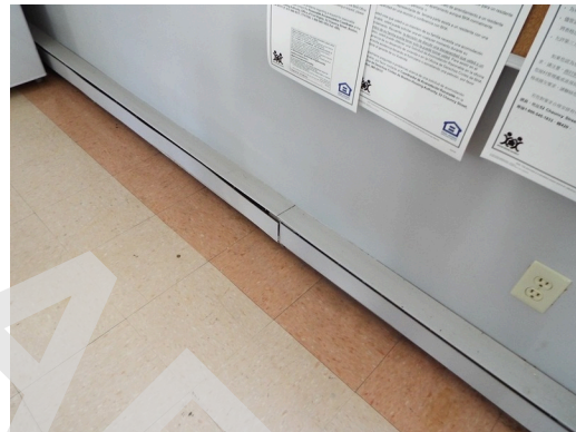
Community building - electric baseboard
