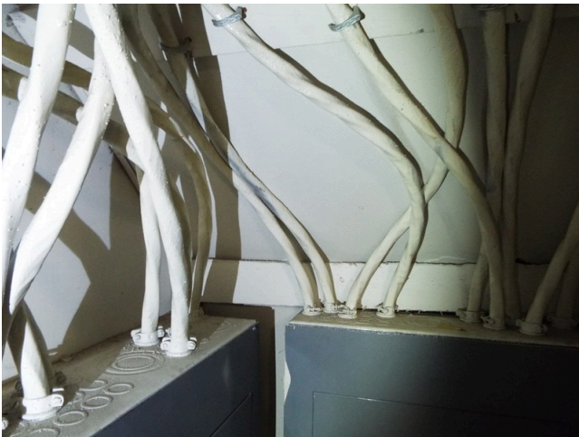
67. Electrical room - building 93-95
