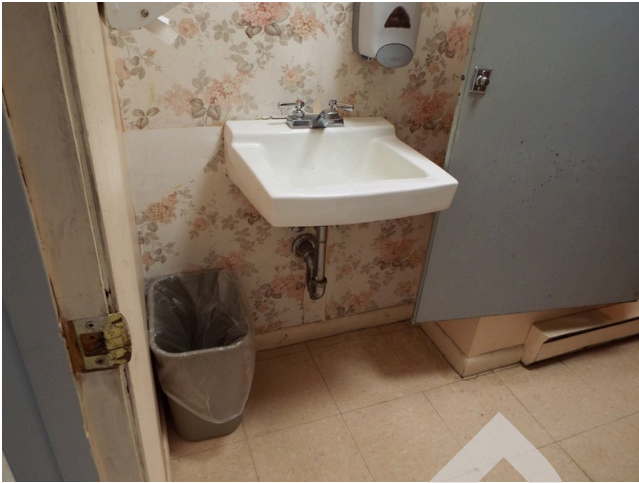
61. Community building - mens room sink lacks pipe protection (Critical Repair)
