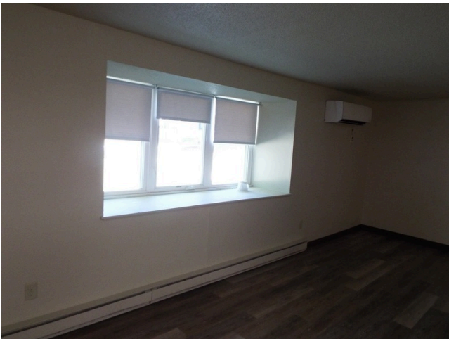
143. Unit electric baseboard (emergency use)
