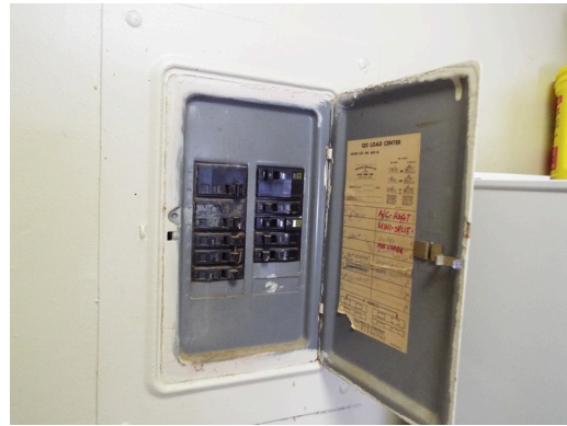
Typical unit electrical panel
