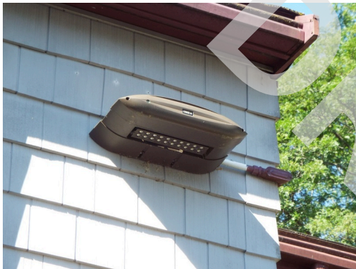
Building mounted lighting
