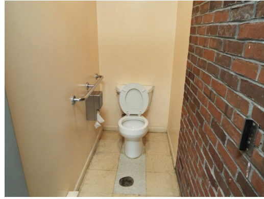
Community building - mens room toilet stall lacks rear grab bar (Critical Repair)
