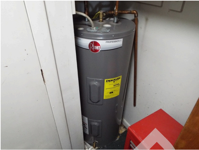
41. 2-bed-1-bath - unit 7 - building 93-95 - water heater
