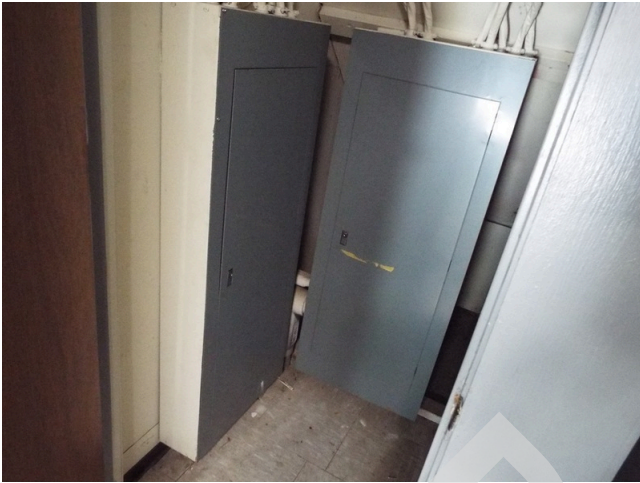
81. Electrical room - building 105-109
