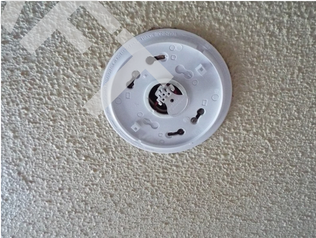
120. 1-bed-1-bath - unit 32 - building 105-109 - typical hardwired smoke detector
