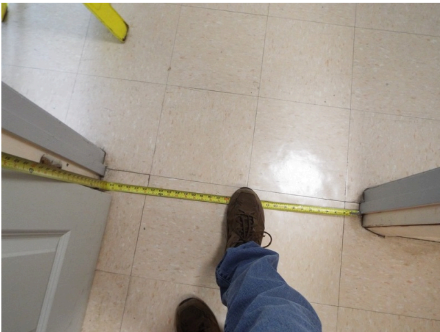
59. Community building - mens room door lacks minum 32 inch clearance (Critical Repair)
