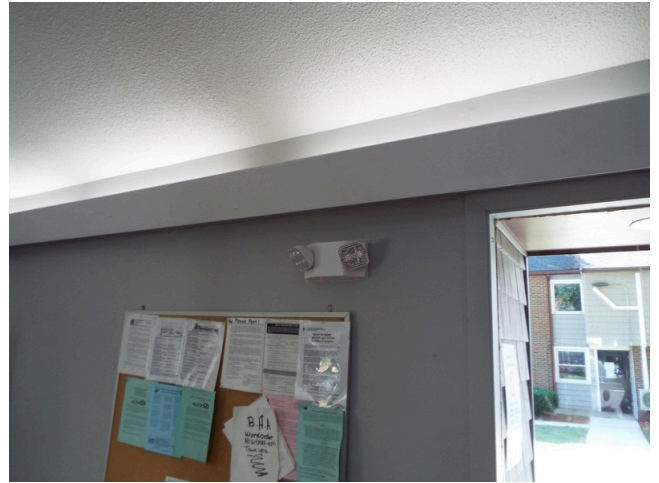
102. Community building - emergency lights
