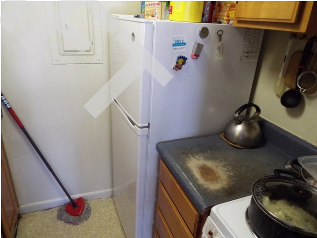
116. 1-bed-1-bath - unit 32 - building 105-109 - countertop condition (Non-Critical Repair)
