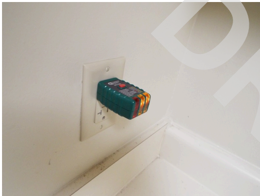
Kitchen GFCI operates correctly
