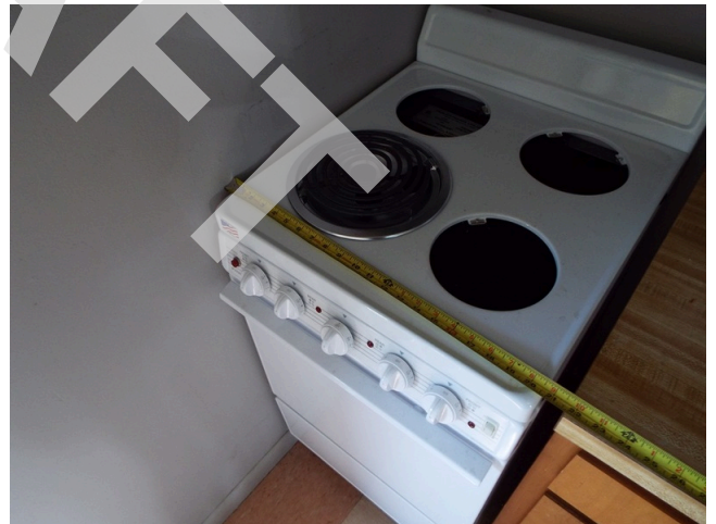
64. Community building - range lacks 30 inch front approach (Critical Repair)
