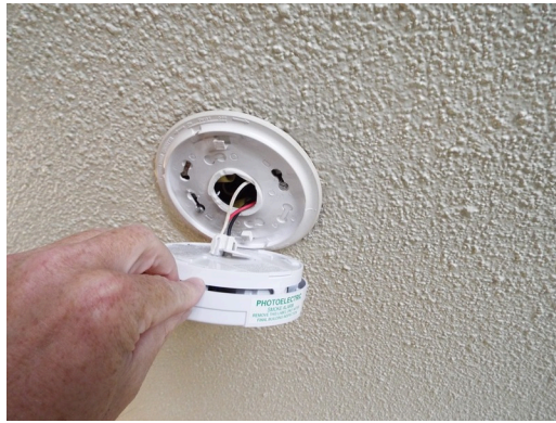
Typical unit hardwired smoke detector
