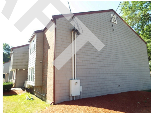
Building electrical service and meter
