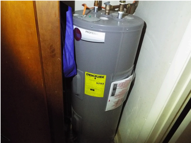
35. 1-bed-1-bath - unit 12 - building 93-95 - water heater
