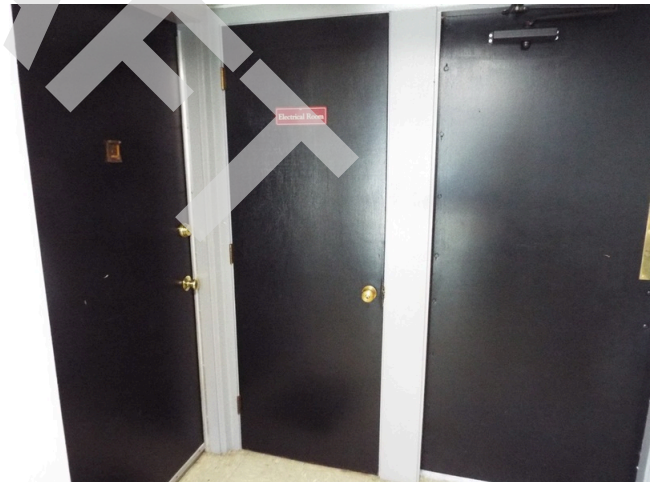
80. Electrical room - building 105-109
