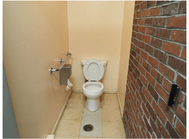
62. Community building - mens room toilet stall lacks rear grab bar (Critical Repair)
