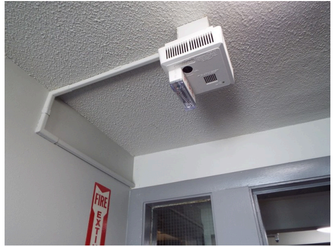
46. Building hallway strobe alarm
