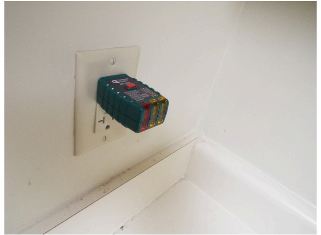
186. Kitchen GFCI operates correctly
