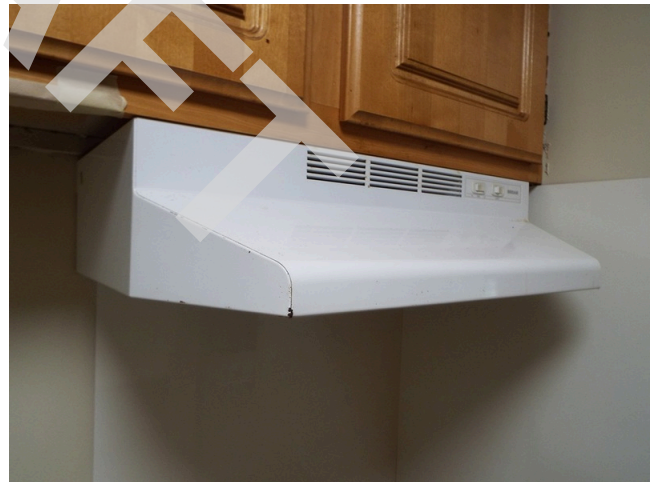
160. 0-bed-1-bath - unit 41 - building 110-112 - range hood
