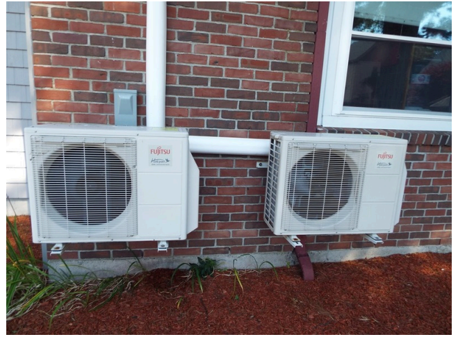
38. Typical mini-split heat pumps
