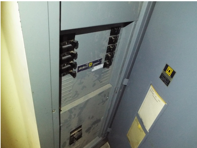
83. Building electrical panel - building 105-109
