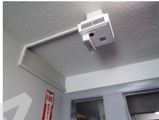
Building hallway strobe alarm
