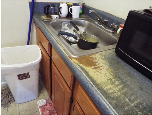
0-bed-1-bath - unit 13 - building 93-95 - countertop condition (Non-Critical Repair)
