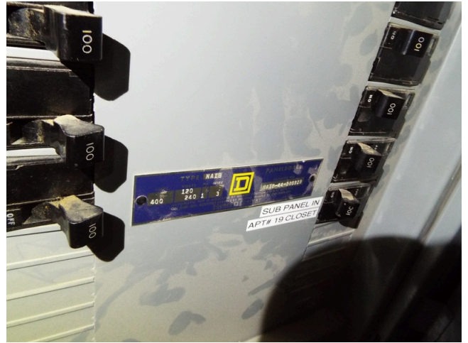
82. Electrical room - building 105-109
