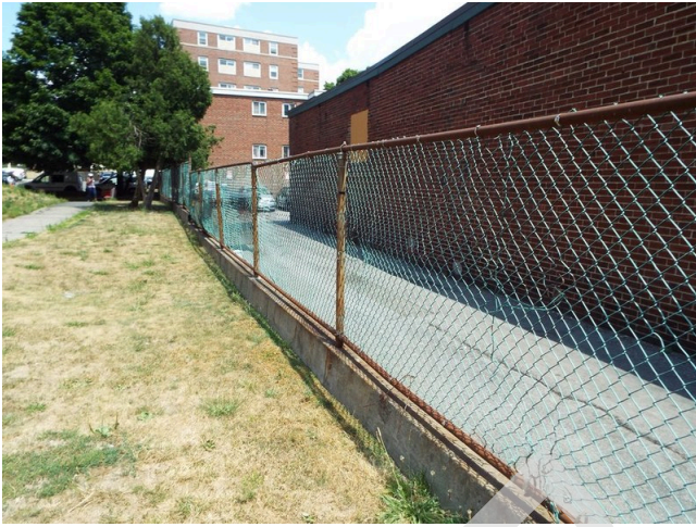
21. Fencing condition (Non-Critical Repair)
