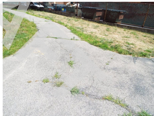
Asphalt walkway condition (Non-Critical Repair)
