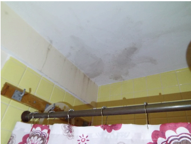
139. 2-bed-1-bath - unit 17 - ceiling condition (Non-Critical Repair)
