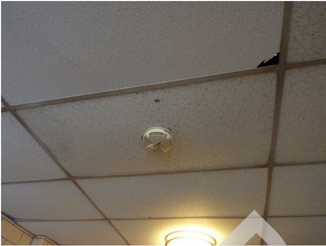
73. Common area smoke detector
