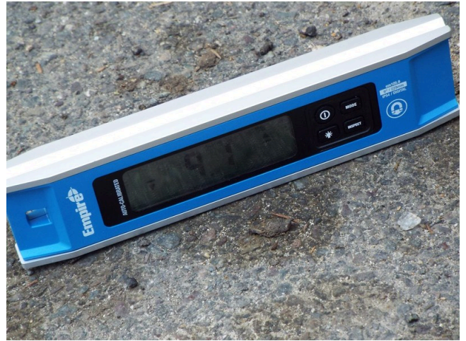
98. Accessible parking - running slope exceeds allowable (Critical Repair)
