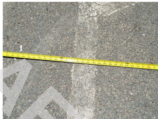
Pavement and striping condition (Non-Critical Repair)
