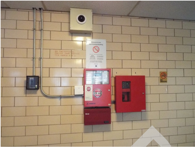
193. Fire alarm control panel
