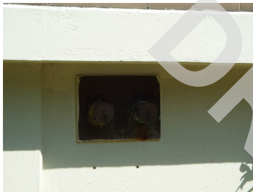
Fire department connection
