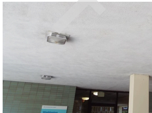
Soffit mounted lighting
