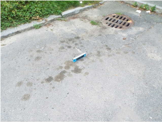
97. Accessible parking - running slope exceeds allowable (Critical Repair)
