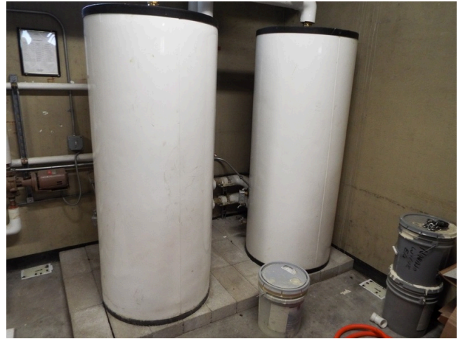
62. Hot water storage tanks
