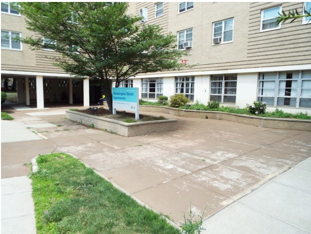
11. Concrete plaza, cracks/deteriorated stain (Non-Critical Repair)
