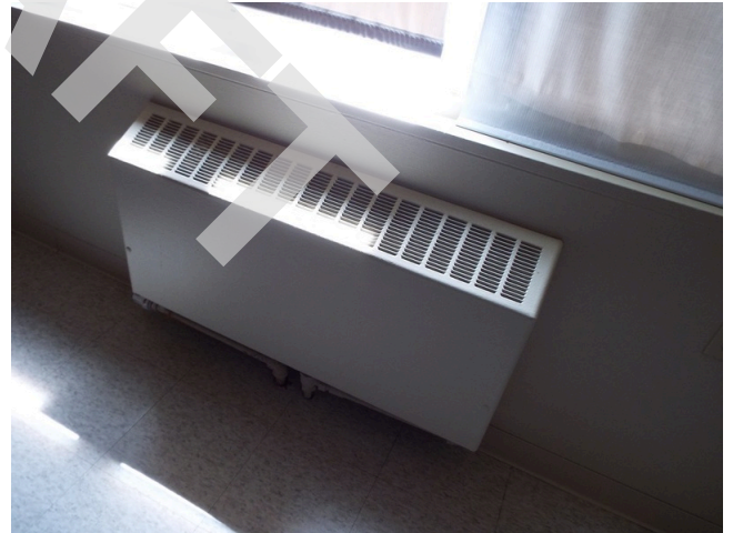
20. 1-bed-1-bath - unit 25 - heating unit
