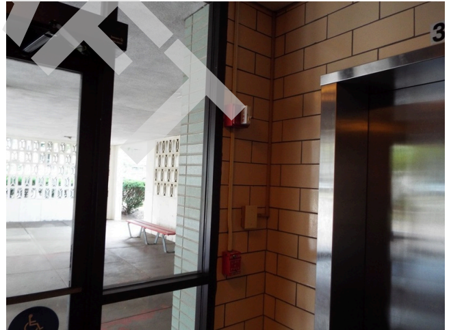
76. Fire life safety devices
