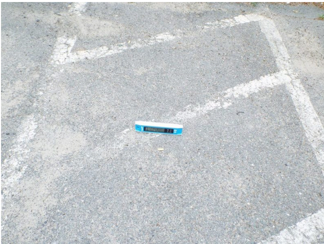
95. Accessible parking - cross slope exceeds allowable (Critical Repair)
