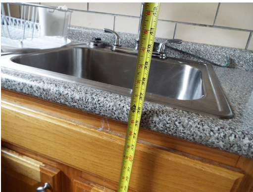
Common area - kitchen sink exceeds 34 inch maximum height
