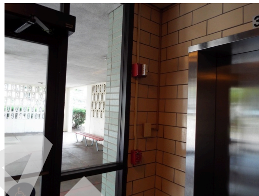
Fire life safety devices
