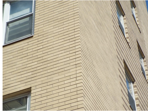
Vertical brick cracking - 91 wing (Non-Critical Repair)
