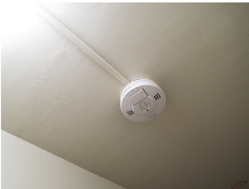
1-bed-1-bath - unit 25 - unit hall way smoke detector
