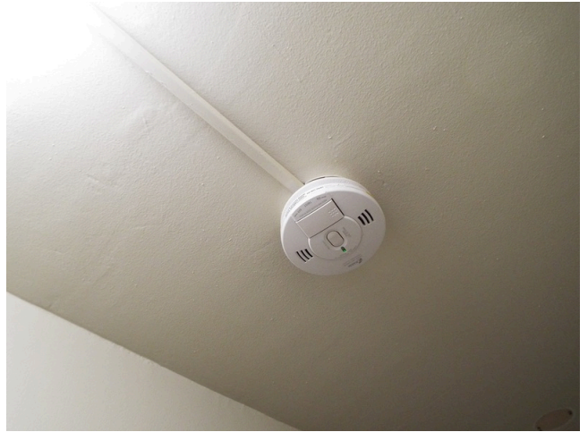
34. 1-bed-1-bath - unit 25 - unit hall way smoke detector
