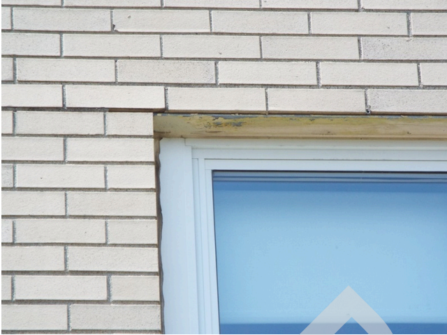
33. Horizontal brick displacement (Non-Critical Repair)
