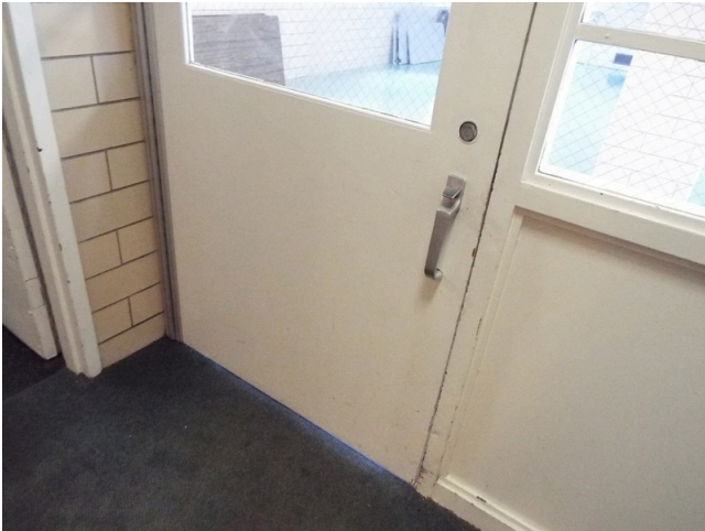
91. Common area - community room non-compliant thumbblatch hardware (Critical Repair)
