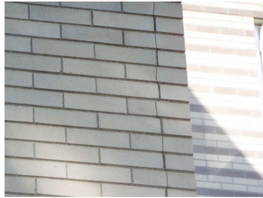
Vertical exterior cracking - 95 wing
