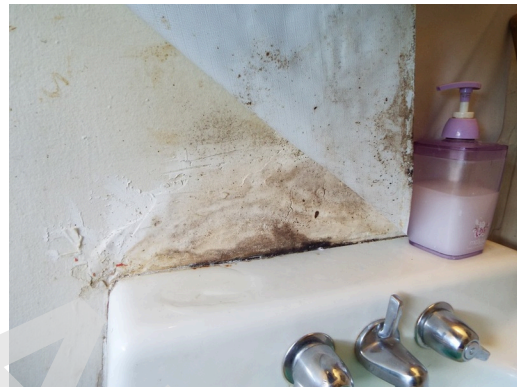
1-bed-1-bath - unit 36 - moisture condition (Critical Repair)
