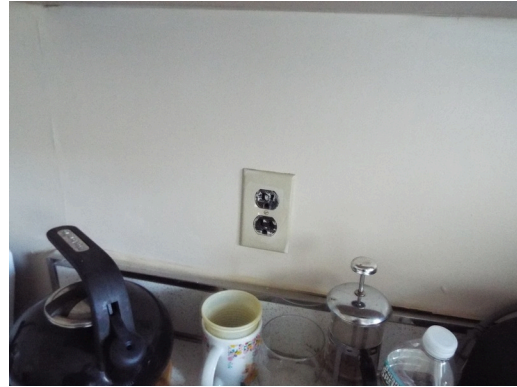
1-bed-1-bath - unit 13 - kitchen lacks GFCI receptacle (Critical Repair)
