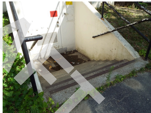
Concrete retaining wall at exterior steps, should sand and paint handrails (Non-Critical Repair)
