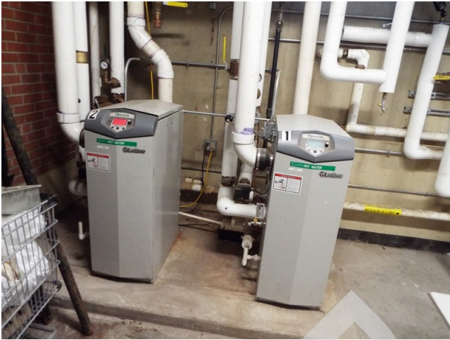
61. Domestic hot water boilers
