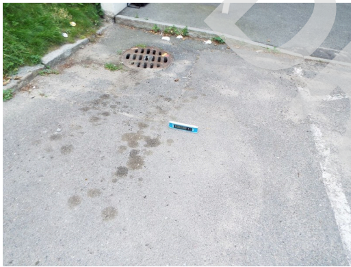
Accessible parking - cross slope exceeds allowable (Critical Repair)
