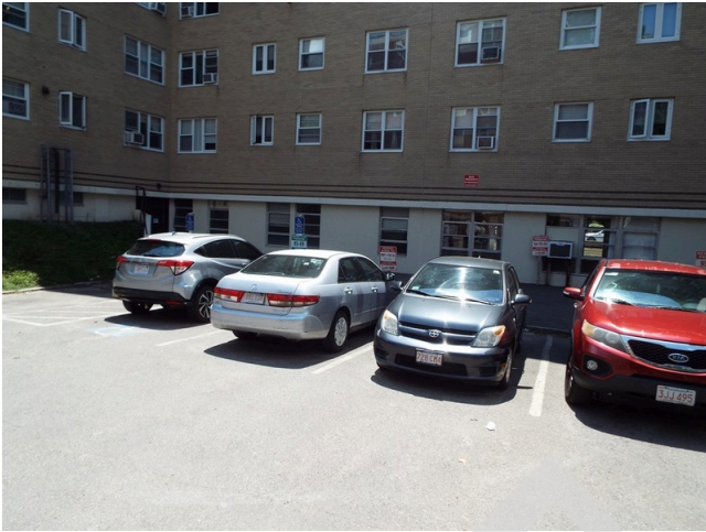
9. Seal coat and striping condition (Non-Critical Repair)
