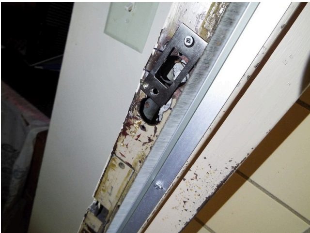
91. 1-bed-1-bath - unit 40 - door lock condition (Critical Repair)
