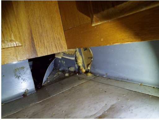
1-bed-1-bath - unit 60 - rodent entry area (Critical Repair)
