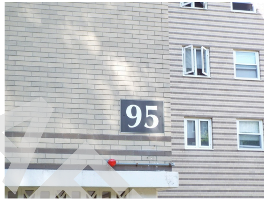
Vertical exterior cracking - 95 wing
