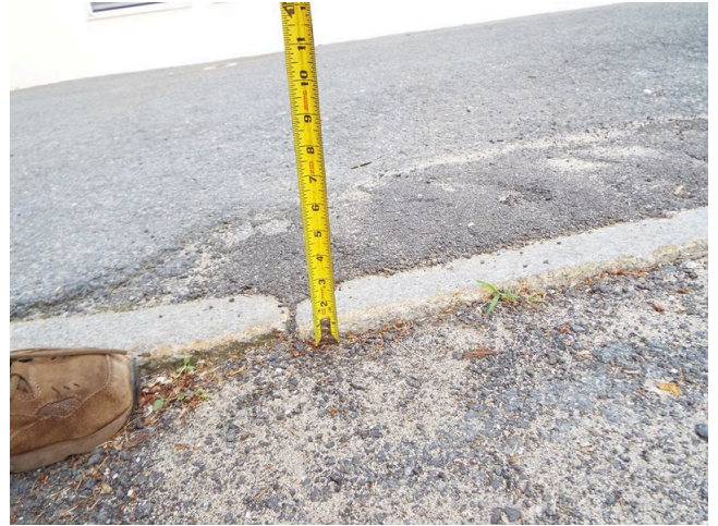
18. Trip hazard - accessible parking access aisle (Critical Repair)
