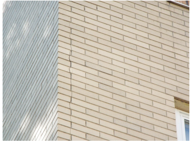
38. Vertical exterior cracking - 95 wing
