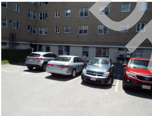
Seal coat and striping condition (Non-Critical Repair)
