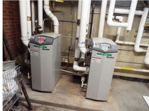
Domestic hot water boilers
