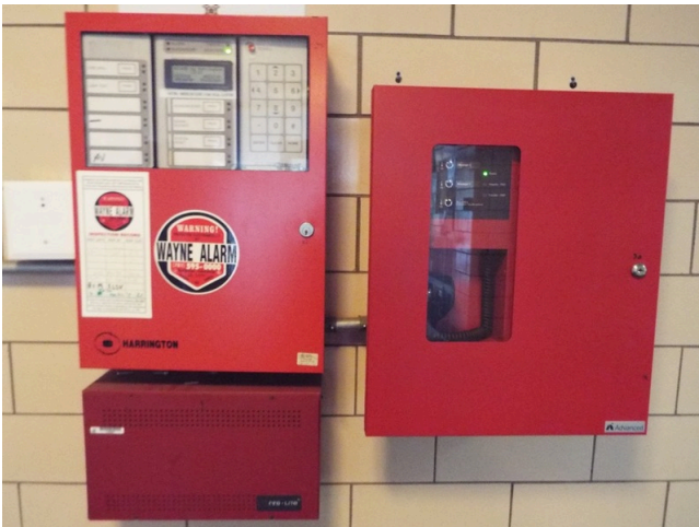
71. Fire alarm control panel
