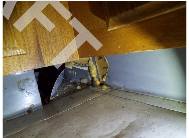
104. 1-bed-1-bath - unit 60 - rodent entry area (Critical Repair)
