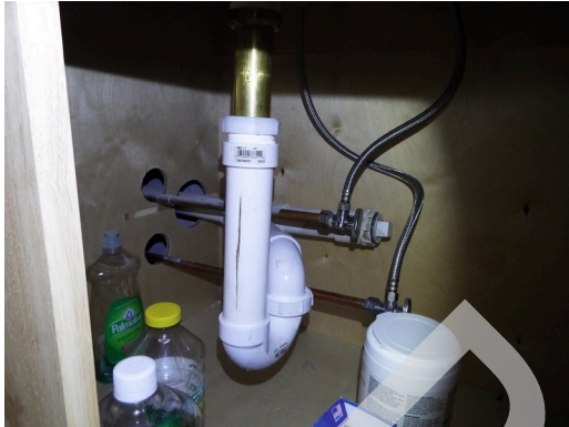
1-bed-1-bath - unit 25 - unit supply and waste piping
