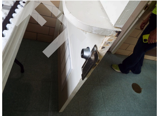
92. Common area - kitchen door lacks lever hardware (Critical Repair)
