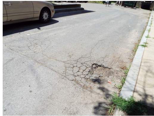
Rear access drive - pavement condition (Non-Critical Repair)
