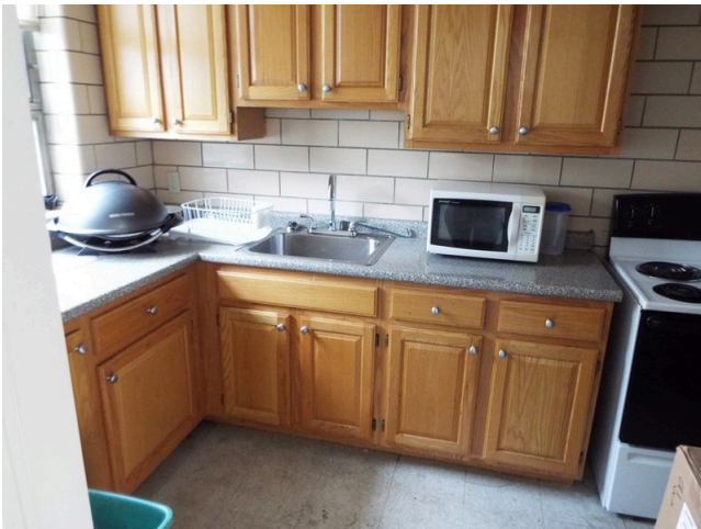
79. Common area - kitchen, not UFAS compliant (Critical Repair)
