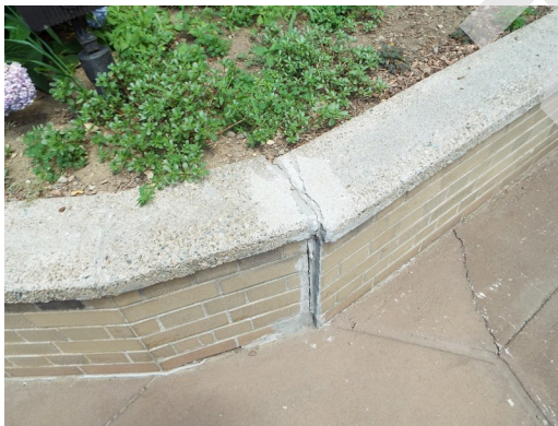
Landscape retaining wall condition (Non-Critical Repair)
