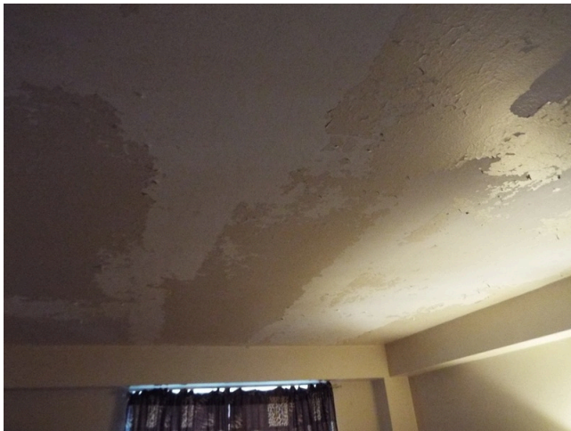
131. 1-bed-1-bath - unit 82 - ceiling paint condition (Non-Critical Repair)
