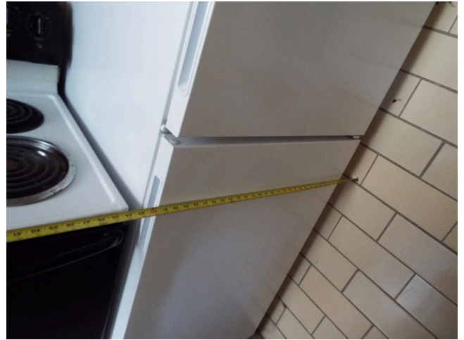
94. Common area - refrigerator lacks 48 inch side access
