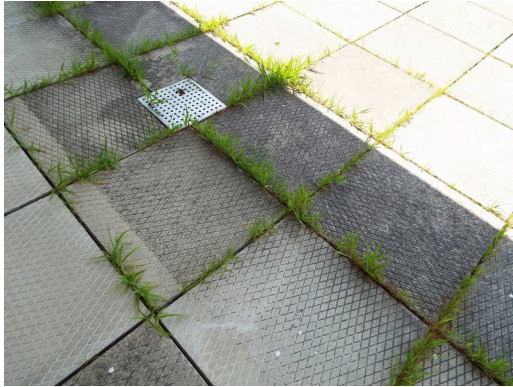
Rooftop terrace vegetation (Non-Critical Repair)
