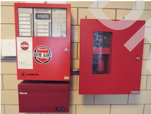
Fire alarm control panel
