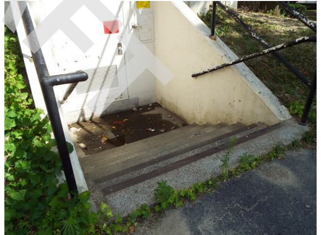
4. Concrete retaining wall at exterior steps, should sand and paint handrails (Non-Critical Repair)
