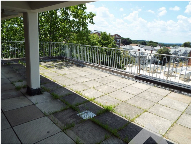
41. Rooftop terrace - 95 wing, treat weeds (Non-Critical Repair)
