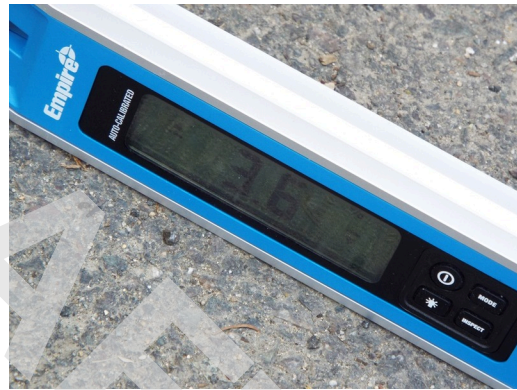
Accessible parking - cross slope exceeds allowable (Critical Repair)
