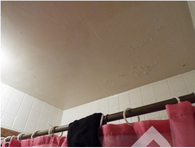
81. 1-bed-1-bath - unit 40 - ceiling paint condition (Non-Critical Repair)
