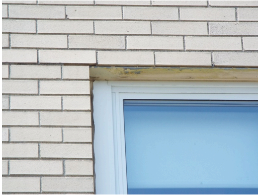
Horizontal brick displacement (Non-Critical Repair)
