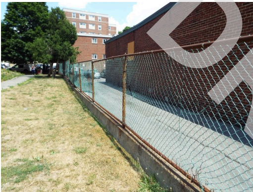
Fencing condition (Non-Critical Repair)
