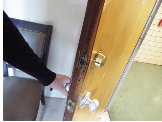
1-bed-1-bath - unit 68 - door lock condition (Critical Repair)
