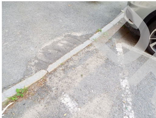
Trip hazard - accessible parking access aisle (Critical Repair)
