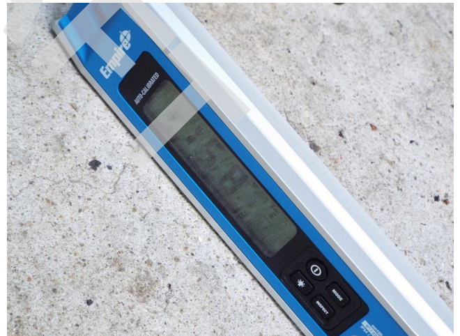
84. Accessible rear entry - slope exceeds allowable (Critical Repair)
