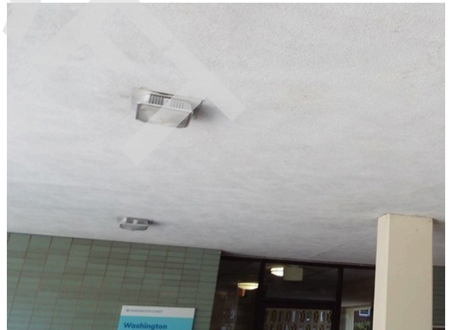
24. Soffit mounted lighting
