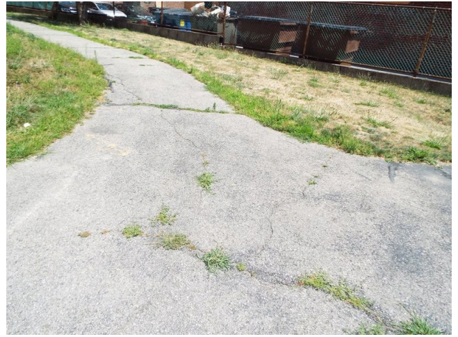
14. Asphalt walkway condition (Non-Critical Repair)
