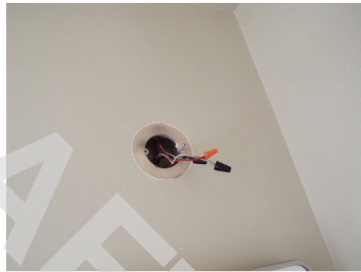
1-bed-1-bath - unit 25 - missing light fixture (Critical Repair)
