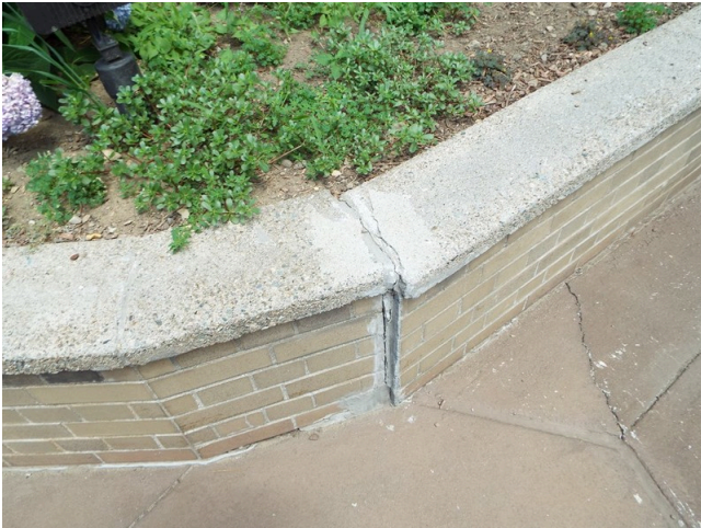
3. Landscape retaining wall condition (Non-Critical Repair)
