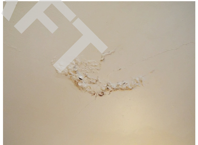
64. 1-bed-1-bath - unit 36 - ceiling condition (Non-Critical Repair)
