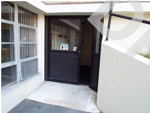
Damaged rear entry door (Critical Repair)
