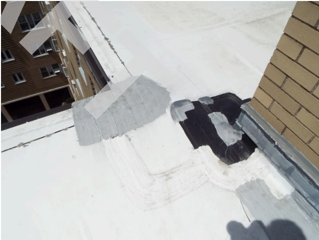
56. Roof flashing (Non-Critical Repair)
