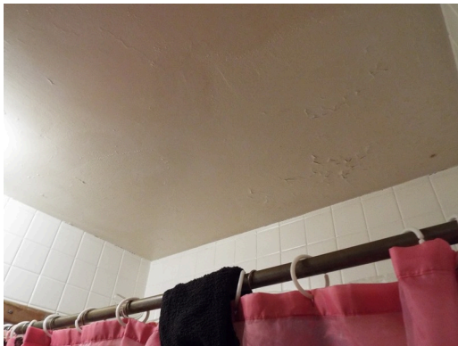
1-bed-1-bath - unit 40 - ceiling paint condition (Non-Critical Repair)
