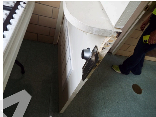
Common area - kitchen door lacks lever hardware (Critical Repair)
