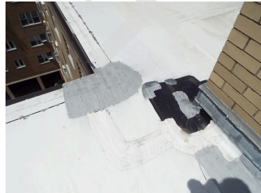
Roof flashing (Non-Critical Repair)
