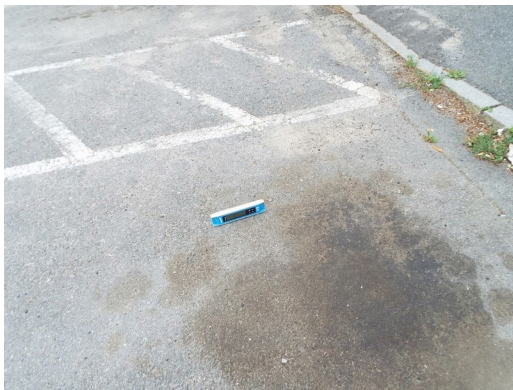
Accessible parking - running slope exceeds allowable (Critical Repair)
