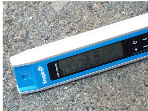
Accessible parking - running slope exceeds allowable (Critical Repair)
