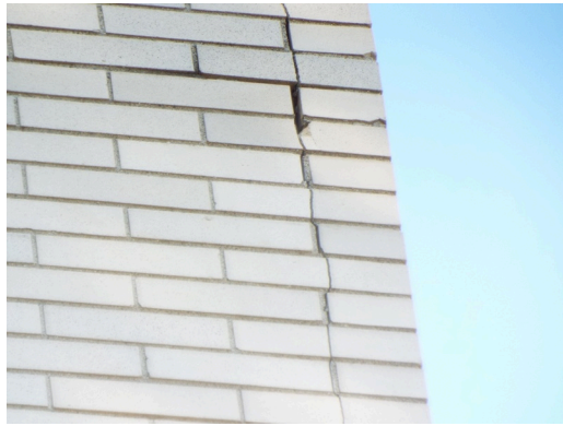
Vertical brick cracking - 95 wing (Non-Critical Repair)
