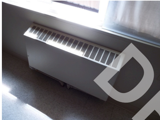
1-bed-1-bath - unit 25 - heating unit
