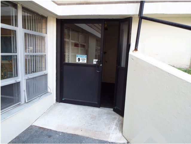
45. Damaged rear entry door (Critical Repair)
