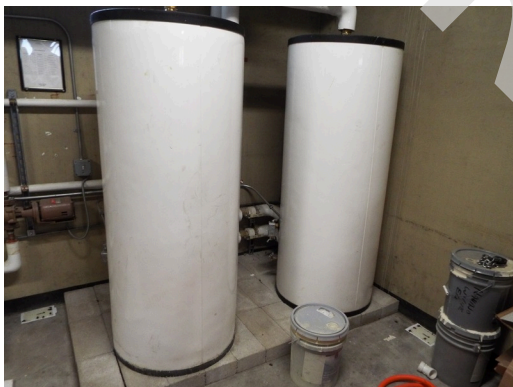
Hot water storage tanks
