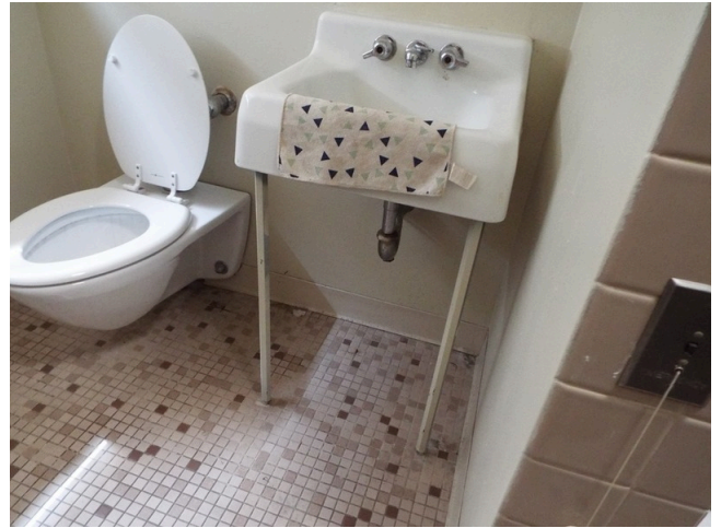
38. 1-bed-1-bath - unit 25 - bathroom fixtures
