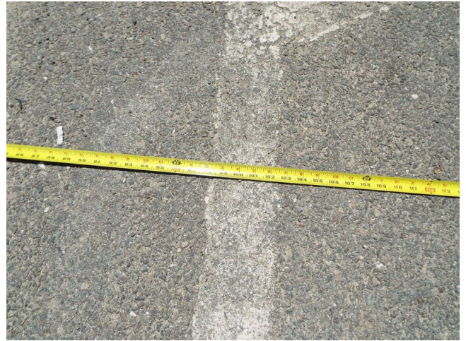
10. Pavement and striping condition (Non-Critical Repair)
