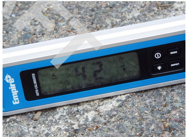
96. Accessible parking - cross slope exceeds allowable (Critical Repair)
