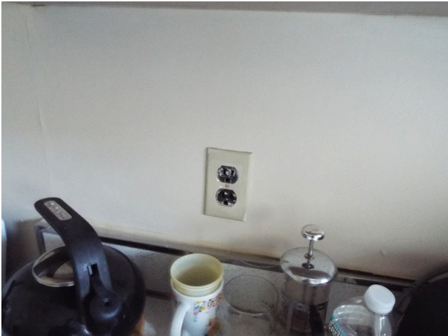
15. 1-bed-1-bath - unit 13 - kitchen lacks GFCI receptacle (Critical Repair)
