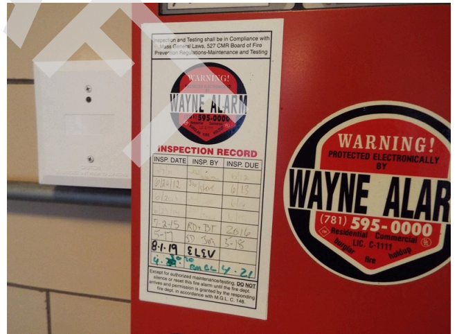
72. Expired fire alarm control panel inspection date (Critical Repair)
