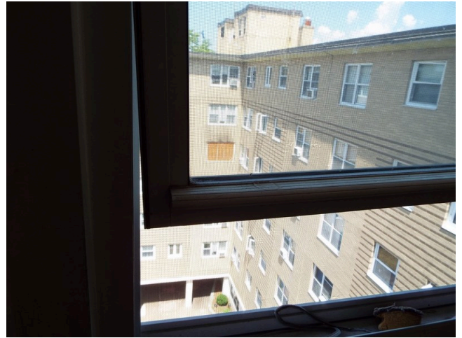
70. 1-bed-1-bath - unit 36 - window condition (Non-Critical Repair)
