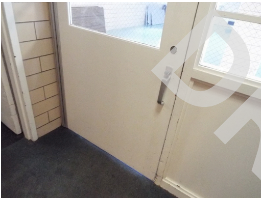
Common area - community room non-compliant thumbblatch hardware (Critical Repair)
