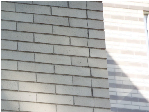
Vertical exterior cracking - 95 wing
