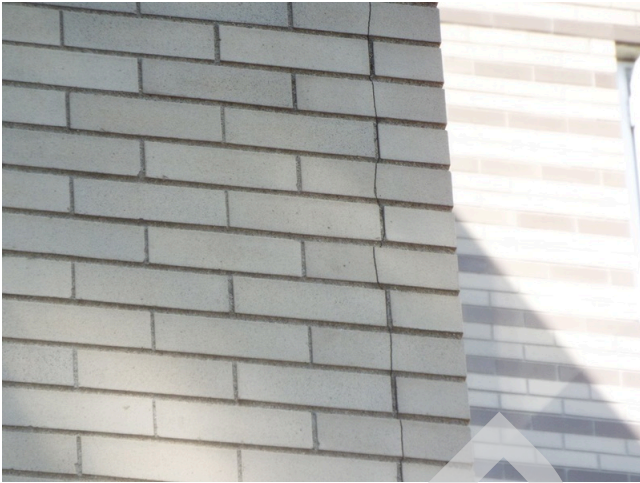
37. Vertical exterior cracking - 95 wing
