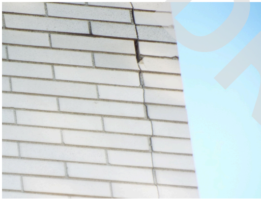
Vertical brick cracking - 95 wing (Non-Critical Repair)
