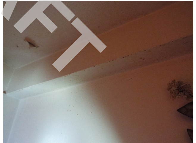
88. 1-bed-1-bath - unit 40 - ceiling paint condition (Non-Critical Repair)
