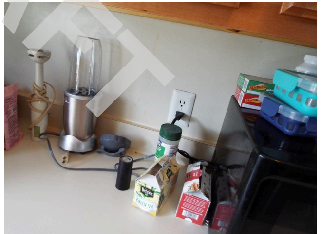
140. 2-bed-1-bath - unit 17 - kitchen lacks GFCI receptacle (Critical Repair)
