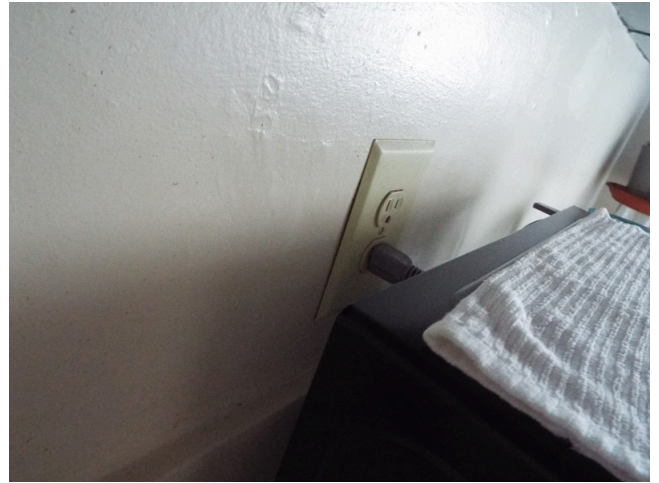
2. 1-bed-1-bath - unit 6 -kitchen lacks GFCI (Critical Repair)
