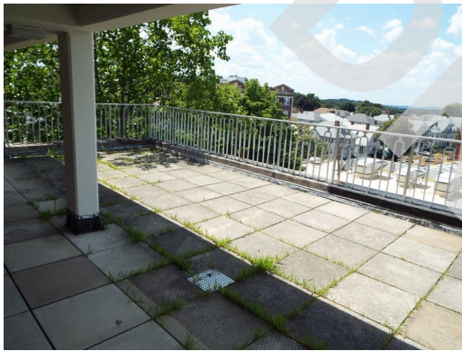
Rooftop terrace - 95 wing, treat weeds (Non-Critical Repair)
