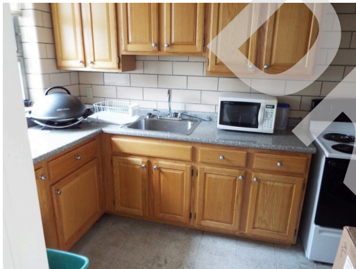
Common area - kitchen, not UFAS compliant (Critical Repair)
