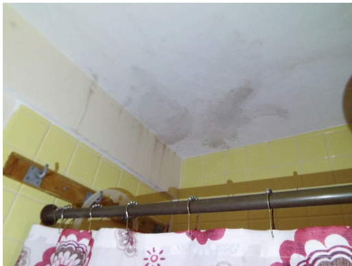
2-bed-1-bath - unit 17 - ceiling condition (Non-Critical Repair)
