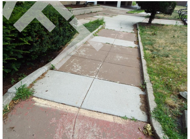
12. Sidewalk condition (Non-Critical Repair)
