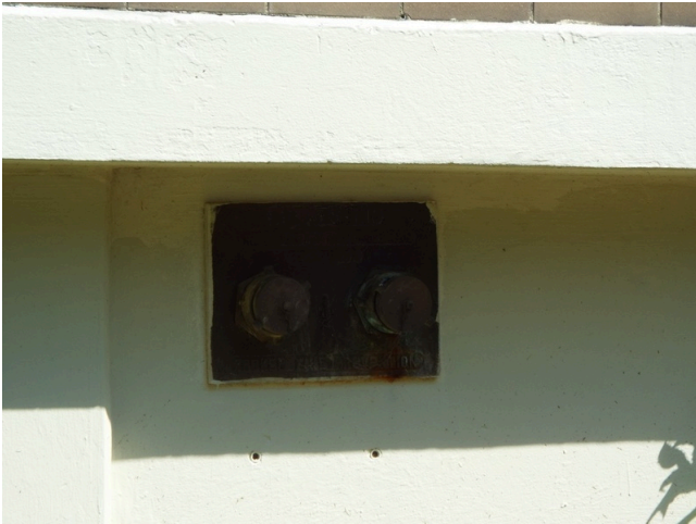
75. Fire department connection
