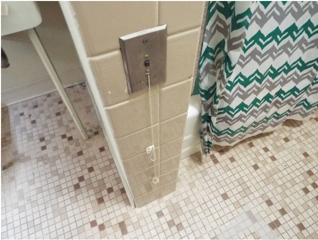
45. 1-bed-1-bath - unit 25 emergency call device (Non-Critical Repair)
