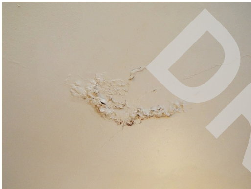
1-bed-1-bath - unit 36 - ceiling condition (Non-Critical Repair)
