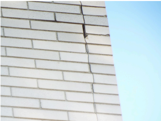
35. Vertical brick cracking - 95 wing (Non-Critical Repair)
