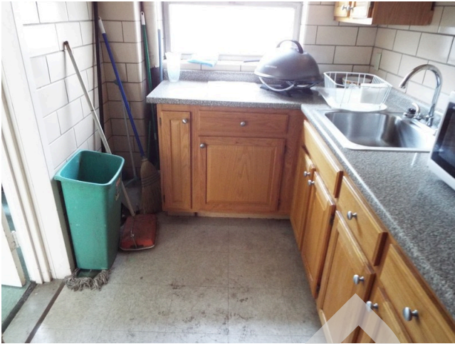
165. Common area - kitchen lacks 60 in turning radius (Critical Repair)
