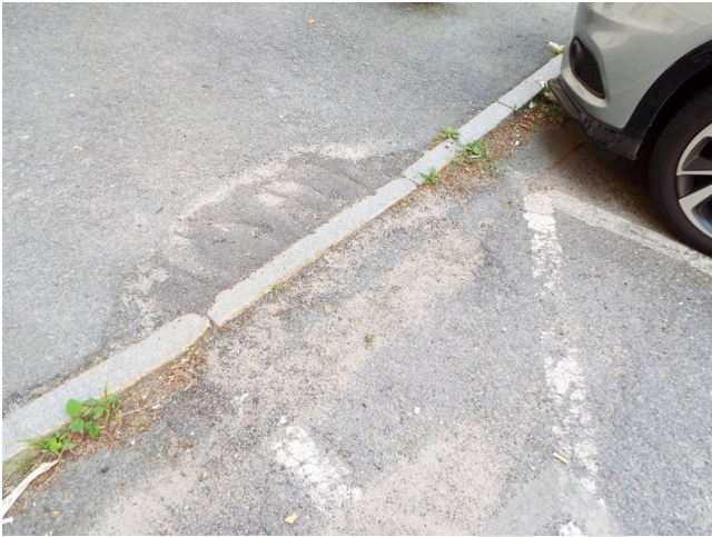
17. Trip hazard - accessible parking access aisle (Critical Repair)
