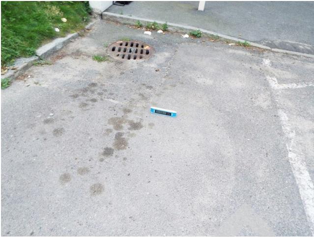
85. Accessible parking - cross slope exceeds allowable (Critical Repair)
