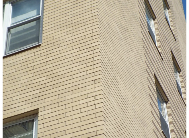
34. Vertical brick cracking - 91 wing (Non-Critical Repair)
