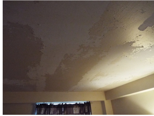
1-bed-1-bath - unit 82 - ceiling paint condition (Non-Critical Repair)
