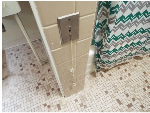
1-bed-1-bath - unit 25 emergency call device (Non-Critical Repair)
