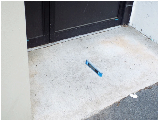
Accessible rear entry - slope exceeds allowable (Critical Repair)
