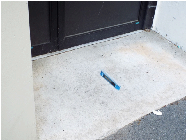
83. Accessible rear entry - slope exceeds allowable (Critical Repair)
