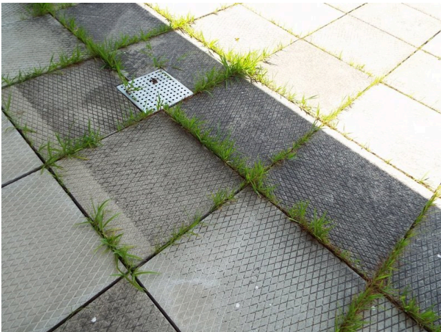
39. Rooftop terrace vegetation (Non-Critical Repair)
