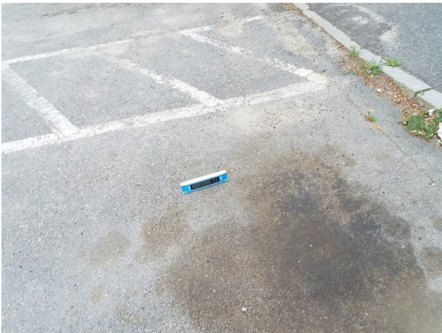
87. Accessible parking - running slope exceeds allowable (Critical Repair)
