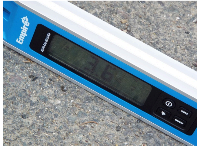
86. Accessible parking - cross slope exceeds allowable (Critical Repair)
