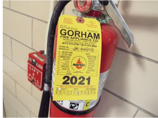
Fire extinguisher - expired service date (Critical Repair)
