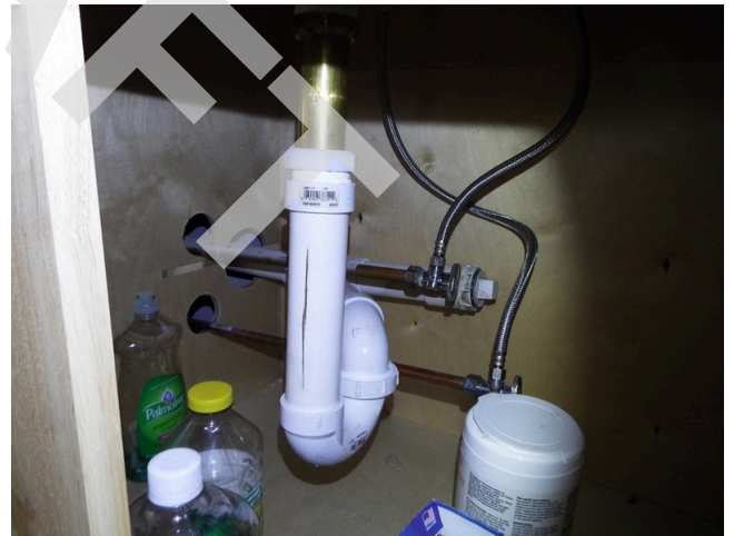
28. 1-bed-1-bath - unit 25 - unit supply and waste piping
