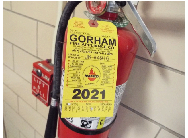
70. Fire extinguisher - expired service date (Critical Repair)
