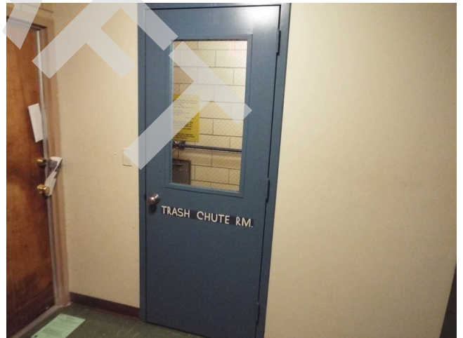
184. Knob hardware at Trash Chute rooms (Critical Repair)
