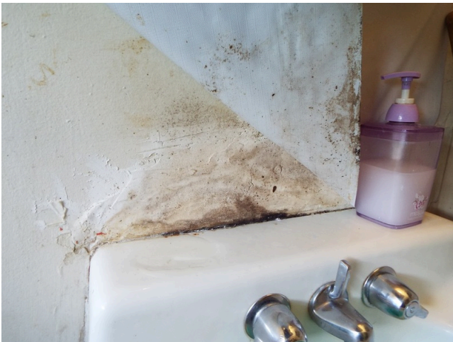
67. 1-bed-1-bath - unit 36 - moisture condition (Critical Repair)
