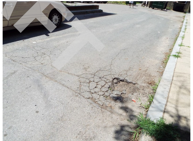
8. Rear access drive - pavement condition (Non-Critical Repair)
