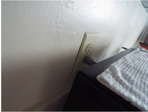
1-bed-1-bath - unit 6 -kitchen lacks GFCI (Critical Repair)
