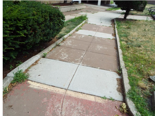
Sidewalk condition (Non-Critical Repair)
