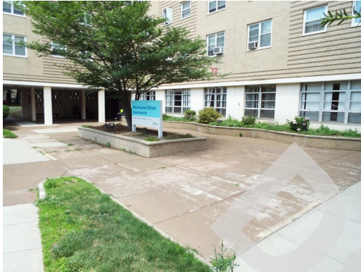
Concrete plaza, cracks/deteriorated stain (Non-Critical Repair)
