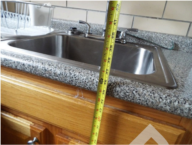
93. Common area - kitchen sink exceeds 34 inch maximum height
