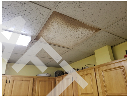
Common Area- Kitchen- Replace Damaged Acoustical Tile Ceiling - Common Area
