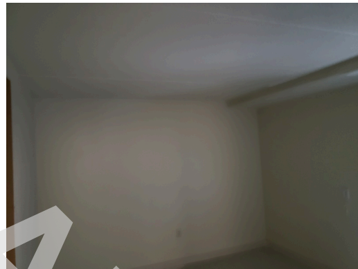
Unit 315- UFAS- 1bed/1bath- Bedroom- Install Bedroom Smoke Detectors Per HUD (Critical Repair)
