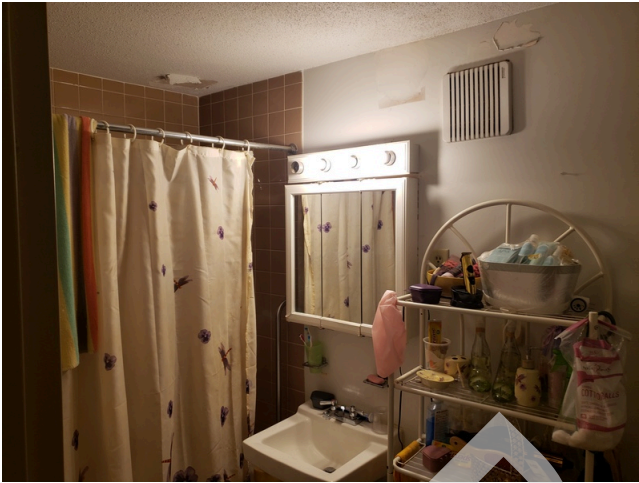
13. Unit 409- 1bed/1bath- Bathroom - Repair Damaged Ceiling (Non-Critical Repair)
