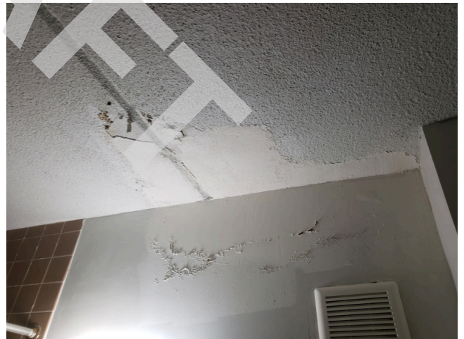
16. Unit 330- 1bed/1bath- Bathroom- Repair Damaged Ceiling (Non-Critical Repair)
