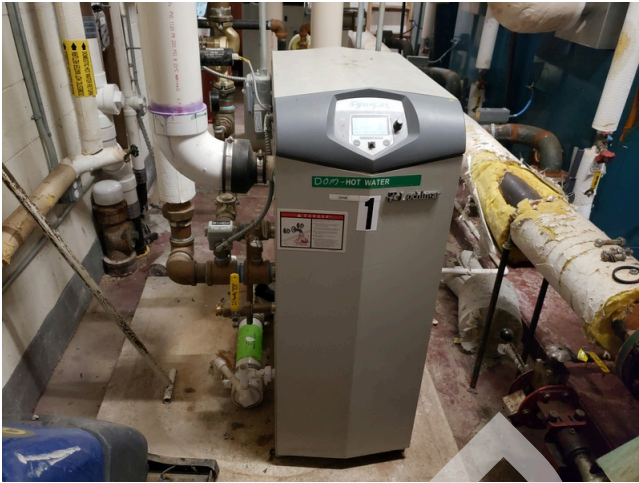
77. Domestic Hot Water Boiler
