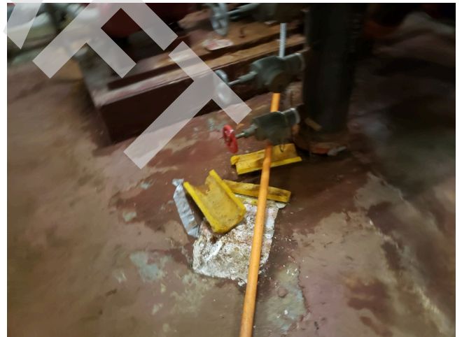
84. Address Leak in Boiler Room (Non-Critical Repair)
