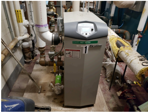
Domestic Hot Water Boiler
