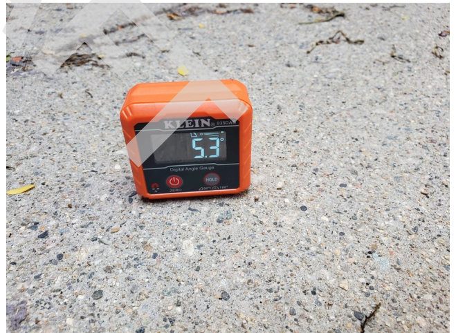
20. Sidewalk Ramp- Install Metal Hand Rail at Ramp (Critical Repair)
