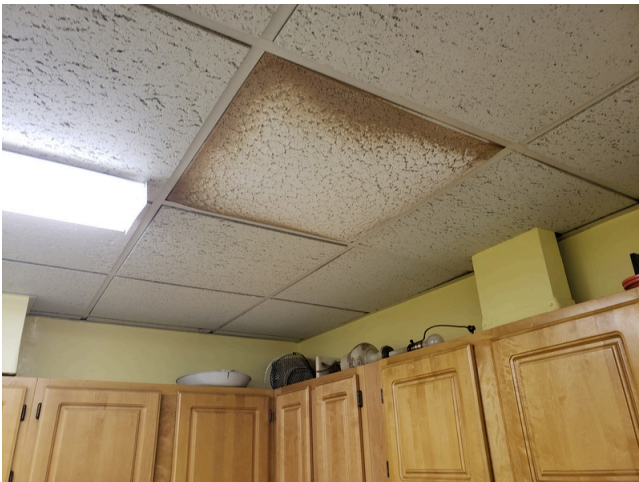
31. Common Area- Kitchen- Replace Damaged Acoustical Tile Ceiling - Common Area
