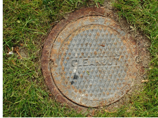
Sewer Clean out
