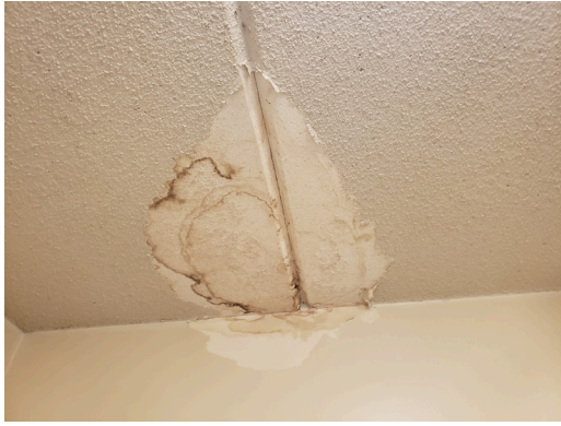
Unit 207- 1bed/1bath- Bathroom- Repair Damaged Ceiling (Non-Critical Repair)
