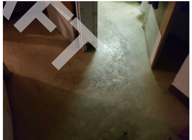
36. Unit 216- UFAS- 1bed/1bath- Replace Vinyl Flooring -1-Bed-Living Room, Kitchens and Baths (Dwelling Units) (Older) (Non-Critical Repair)
