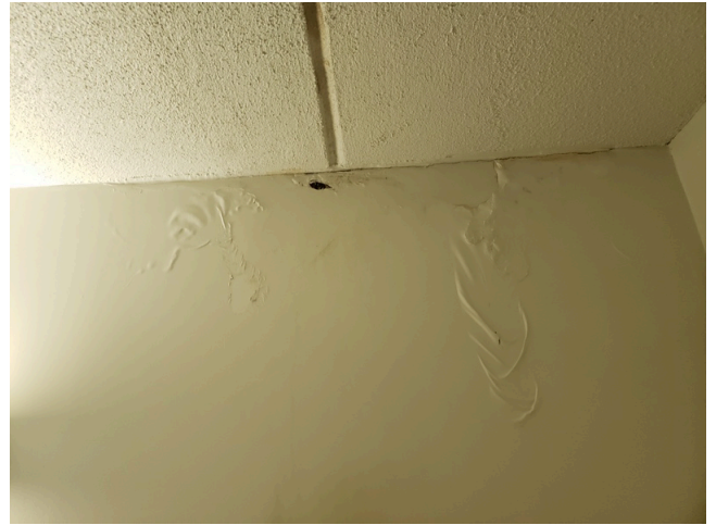
38. Unit 216- UFAS- 1bed/1bath- Bathroom- Repair Damaged Ceiling (Non-Critical Repair)
