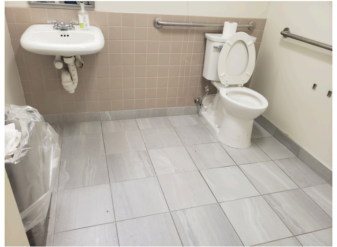
34. Common Area- Public Men's Restroom
