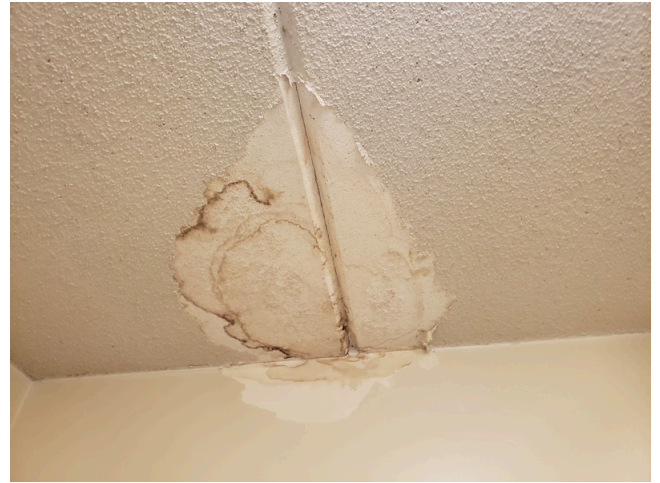
34. Unit 207- 1bed/1bath- Bathroom- Repair Damaged Ceiling (Non-Critical Repair)
