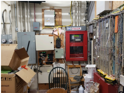
Main Fire Panel
