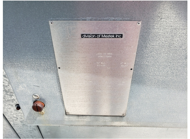
86. Roof-Top Make Up Air Unit (Non-Critical Repair)
