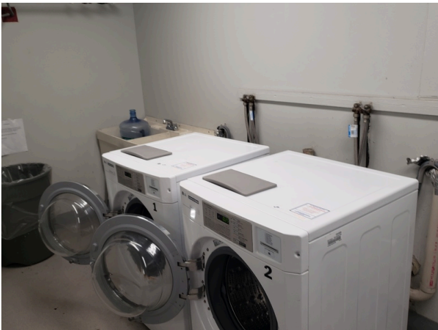
51. Leased Washer/ Dryer w/ Laundry Sink
