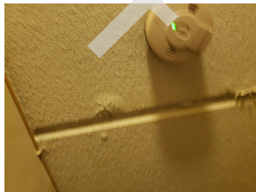
Typical Smoke Detector
