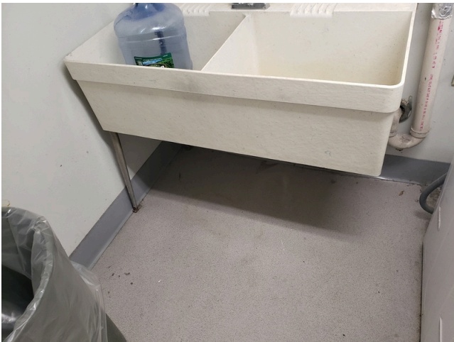
47. Common Area Laundry- Sink
