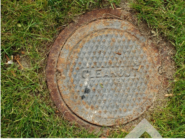
61. Sewer Clean out
