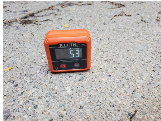
Sidewalk Ramp- Install Metal Hand Rail at Ramp (Critical Repair)
