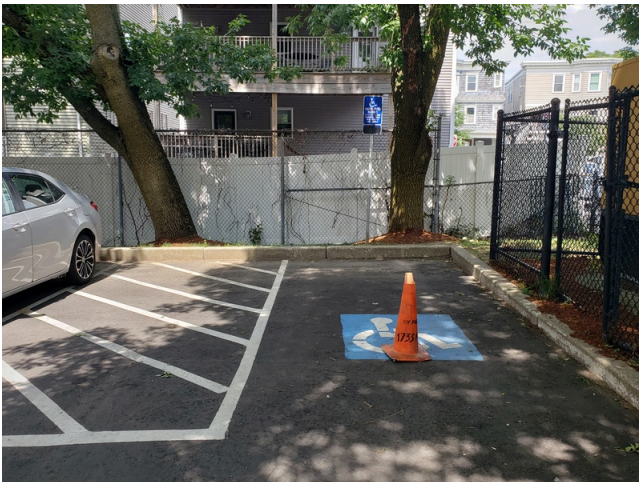
7. ADA Parking Lot- Install Van Accessible Parking Signage (Critical Repair)
