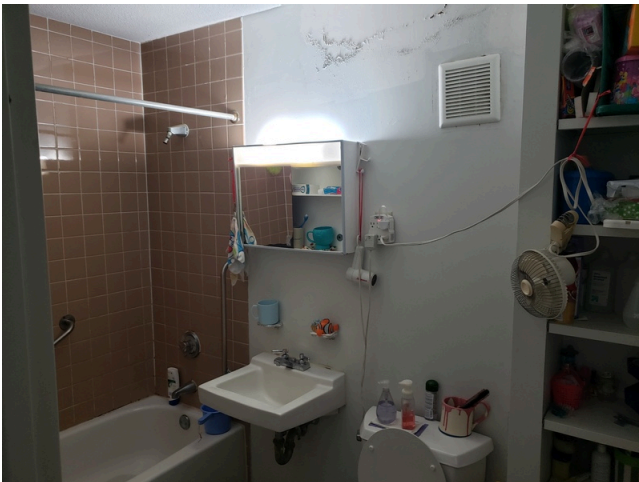
15. Unit 330- 1bed/1bath- Bathroom- Repair Damaged Ceiling (Non-Critical Repair)
