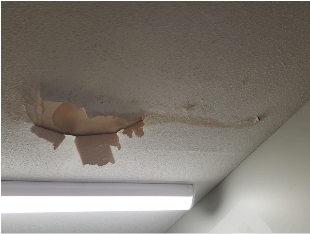
57. Common Area Hallway near Unit 317 - Repair Damaged Ceiling (Non-Critical Repair)
