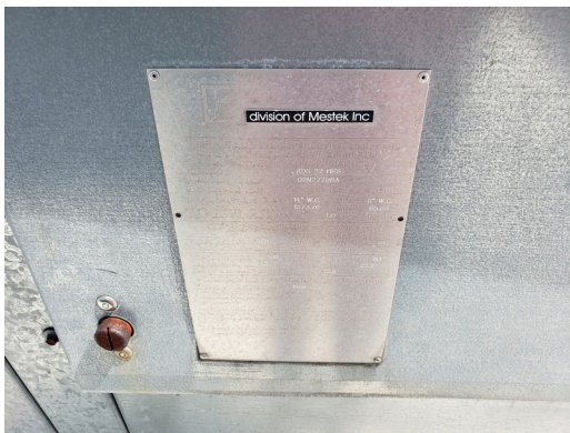
Roof-Top Make Up Air Unit (Non-Critical Repair)
