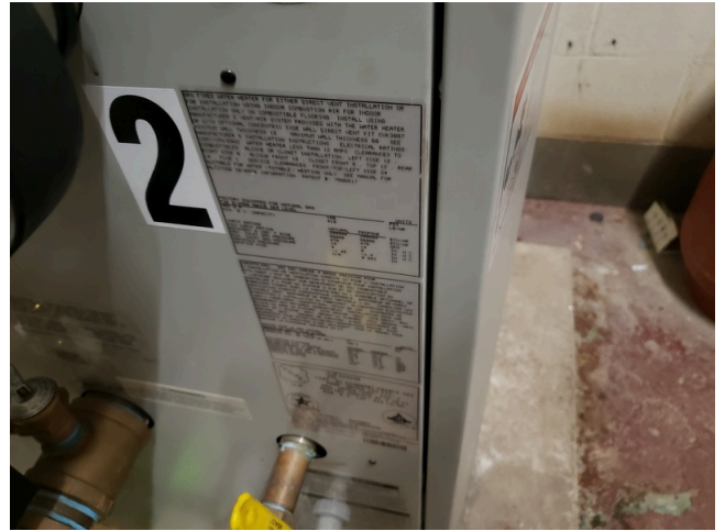
78. Domestic Hot Water Boiler
