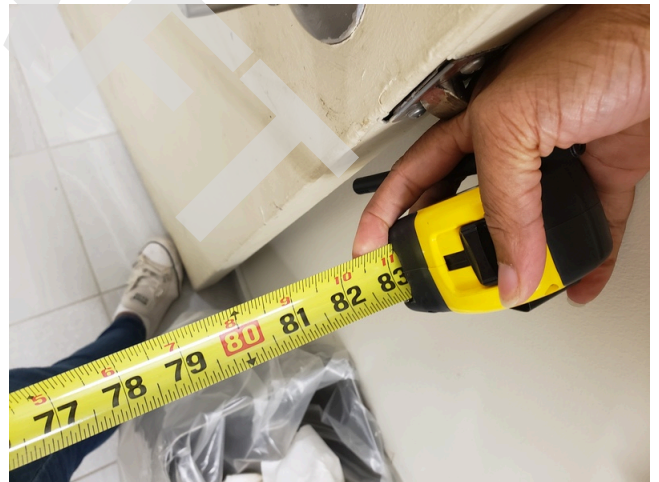
36. Common Area- Public Men's Restroom- Clear Floor Space at Door to Sink
