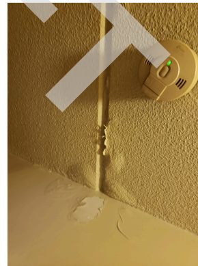
Unit 207- 1bed/1bath- Bathroom- Repair Leak in Hallway- Repair Damaged Ceiling (Non-Critical Repair)
