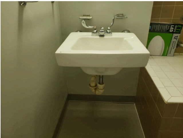
51. Unit 101-UFAS HDCP- 2bed/1bath- Bathroom- Install Scald and Abrasion Sink Wrap (Critical Repair)
