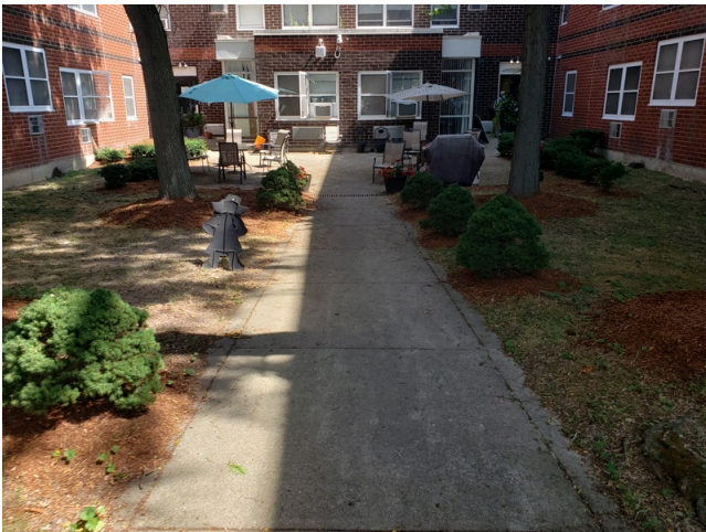
19. Sidewalk Ramp- Install Metal Hand Rail at Ramp (Critical Repair)
