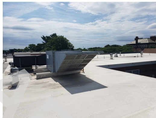
Roof-Top Make Up Air Unit (Non-Critical Repair)
