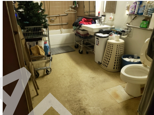
Unit 216- UFAS- 1bed/1bath- Replace Vinyl Flooring -1-Bed-Living Room, Kitchens and Baths (Dwelling Units) (Older) (Non-Critical Repair)
