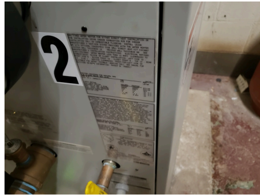
Domestic Hot Water Boiler
