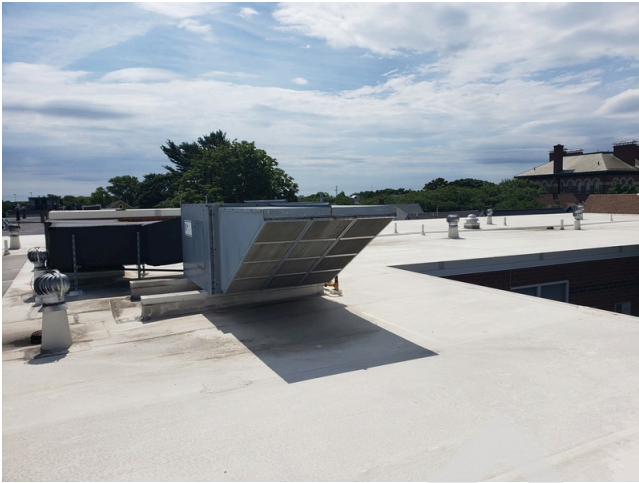
85. Roof-Top Make Up Air Unit (Non-Critical Repair)
