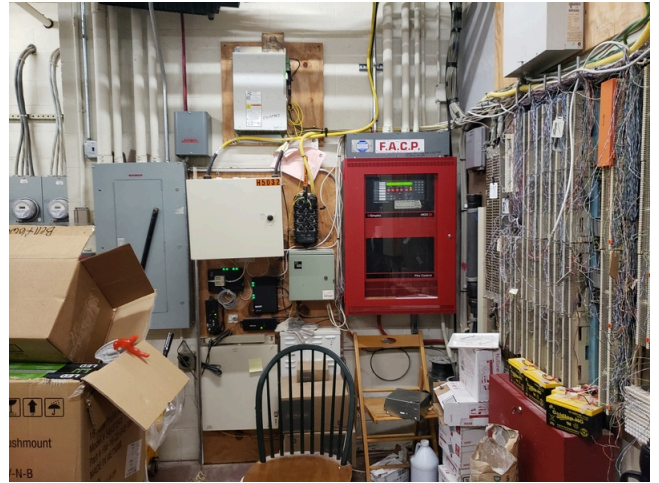
70. Main Fire Panel
