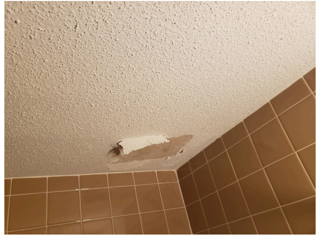
14. Unit 409- 1bed/1bath- Bathroom- Repair Damaged Ceiling (Non-Critical Repair)
