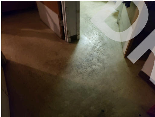
Unit 216- UFAS- 1bed/1bath- Replace Vinyl Flooring -1-Bed-Living Room, Kitchens and Baths (Dwelling Units) (Older) (Non-Critical Repair)
