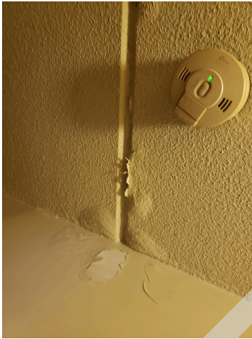
33. Unit 207- 1bed/1bath- Bathroom- Repair Leak in Hallway- Repair Damaged Ceiling (Non-Critical Repair)
