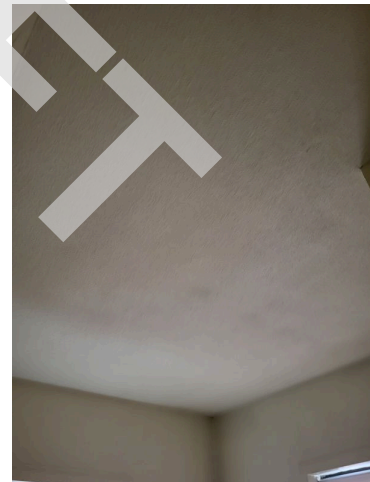
52. Apartment 56-3 bedroom missing smoke detector (Critical Repair)
