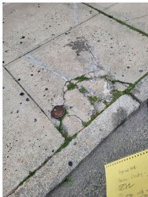
West elevation sidewalk damage trip hazard (Critical Repair)
