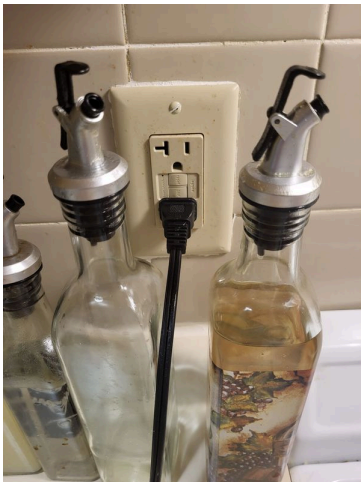
7. Apartment 54-2 kitchen GFCI
