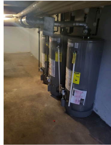
102. Hot water heaters
