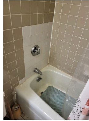
Apartment 56-3 bathroom bathtub hardware
