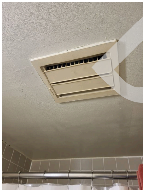
Apartment 56-3 bathroom ventilation
