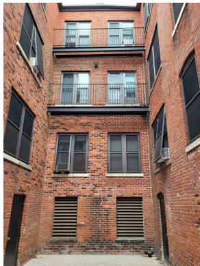
Southeast elevation court yard brick façade, balcony railings, window screens and high density light fixture
