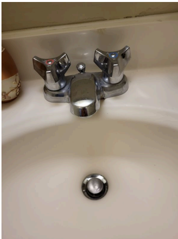
91. Apartment 52-3 bathroom sink faucet
