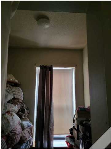
105. Apartment 52-3 bedroom light fixture and missing smoke detector (Critical Repair)
