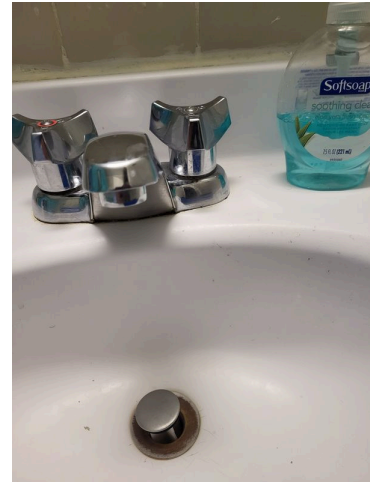
70. Apartment 58-3 bathroom sink faucet
