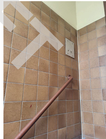
24. Building ingress/egress stairs railing and intercom (Non-Critical Repair)
