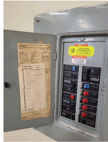
82. Gould electrical Panel
