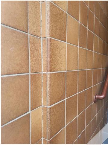
21. Building ingress/egress ceramic tile wall damage (Non-Critical Repair)
