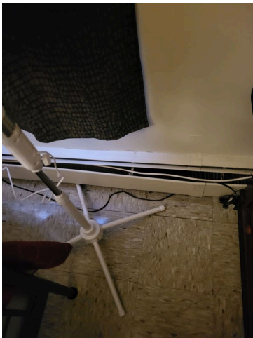
27. Apartment 54-2 bedroom hydronic baseboard (Non-Critical Repair)
