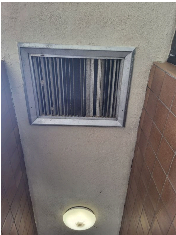
27. Common hallway ventilation
