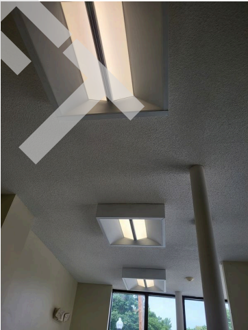
92. Common area hallway light fixtures
