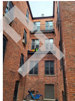
Northeast elevation court yard brick façade, balcony railings, window screens and high density light fixture
