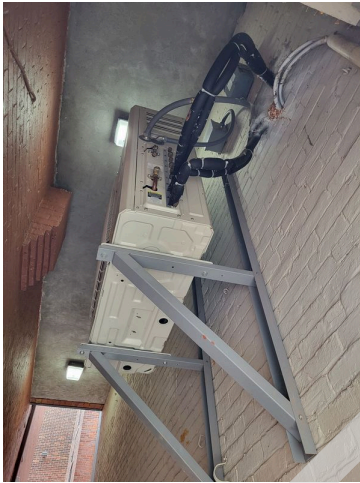
53. Court yard ingress/egress mini split system and light fixtures
