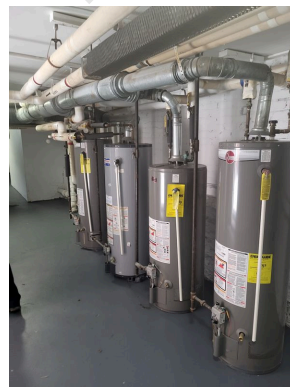
Hot water heater copper pipes
