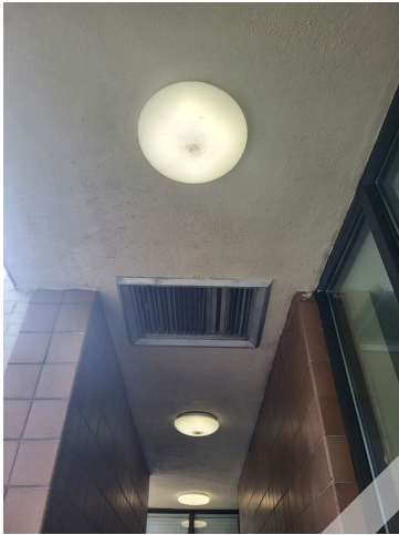
25. Common hallway light fixture
