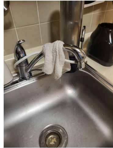
6. Apartment 54-2 kitchen sink and faucet
