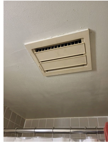
42. Apartment 56-3 bathroom ventilation
