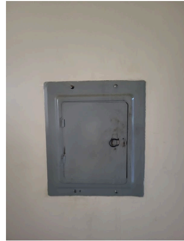
38. Apartment 56-3 circuit breaker box
