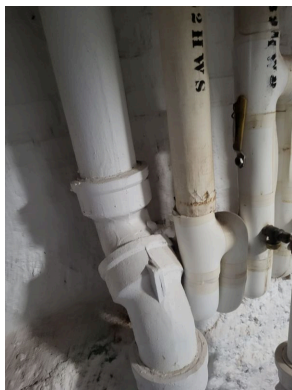
Cast iron pipe
