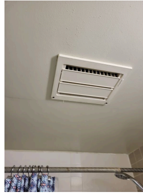
Apartment 54-2 bathroom ventilation
