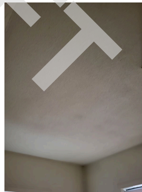
Apartment 56-3 bedroom missing smoke detector (Critical Repair)
