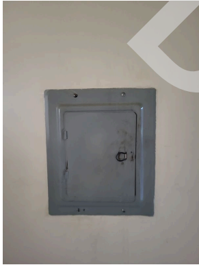
Apartment 56-3 circuit breaker box
