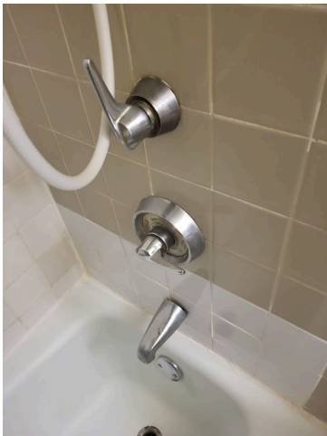
23. Apartment 54-2 bathroom bathtub hardware
