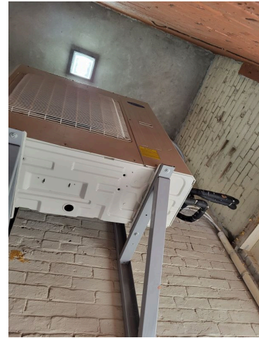
54. Court yard ingress/egress mini split system
