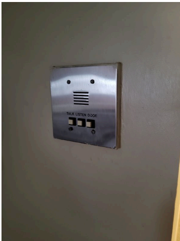
3. Apartment 54-2 intercom (Non-Critical Repair)
