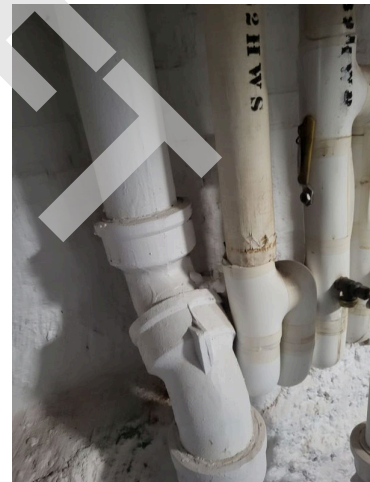
112. Cast iron pipe
