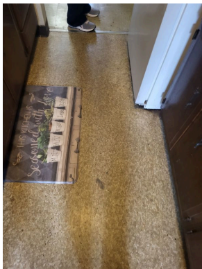
Apartment 56-3 kitchen sheet vinyl flooring (Non-Critical Repair)
