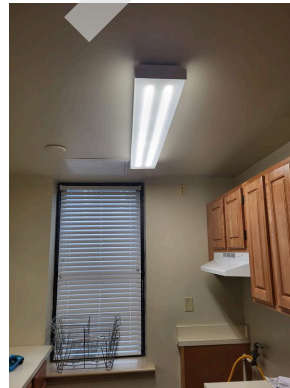
Community room kitchen area light fixture
