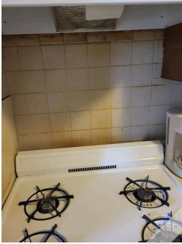
29. Apartment 56-3 kitchen range and range hood
