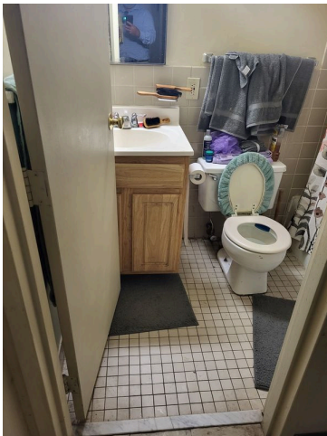
39. Apartment 56-3 bathroom vanity, sink, toilet and flooring
