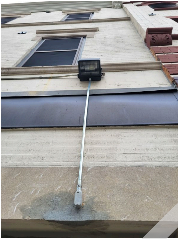
49. Exterior wall mounted high density light fixture
