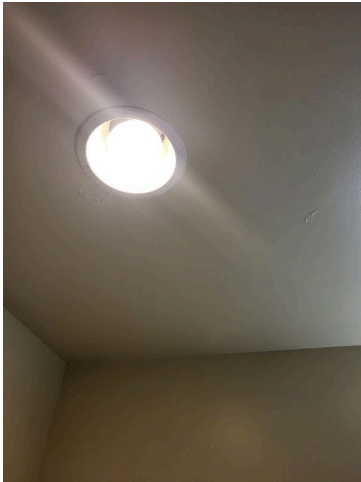
91. Community room restroom light fixture
