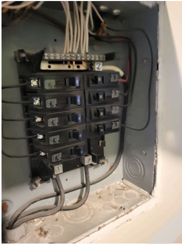
73. Apartment 58-3 circuit breaker box (Critical Repair)
