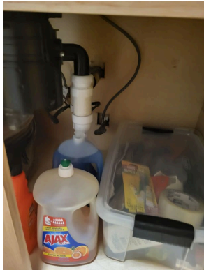
Apartment 54-2 kitchen garbage disposal
