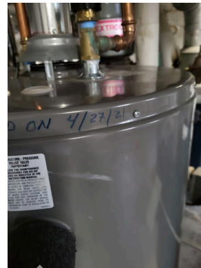
Hot water heater
