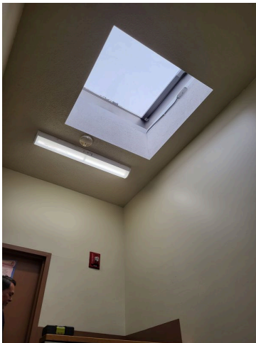
55. Common area stairwell sky light, light fixture and smoke detector
