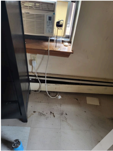
53. Apartment 56-3 bedroom hydronic baseboard damage (Non-Critical Repair)
