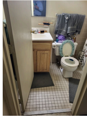
Apartment 56-3 bathroom vanity, sink, toilet and flooring
