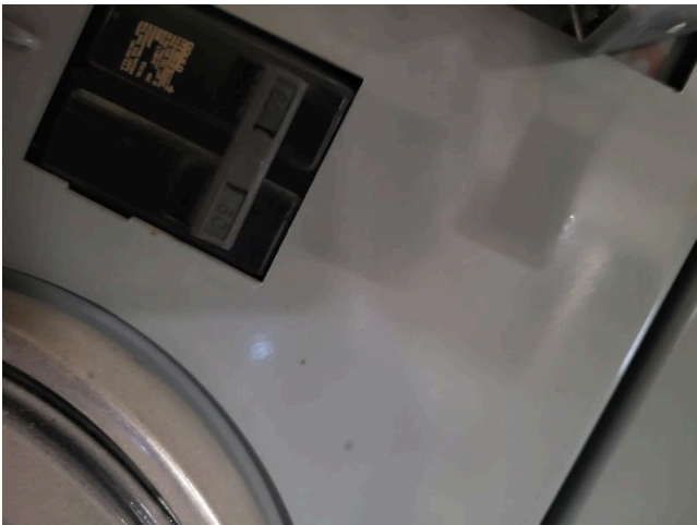
115. Gould main breaker switch
