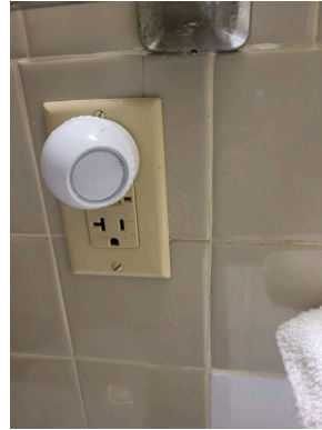
Apartment 54-2 bathroom GFCI
