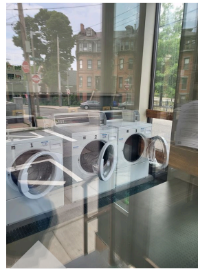
Common area laundry room front end loader washers
