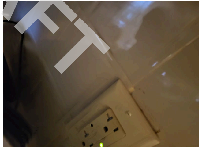
84. Apartment 52-3 kitchen GFCI
