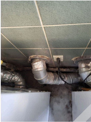
93. Laundry room dryer vent damaged (Non-Critical Repair)
