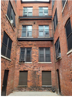
Southeast elevation court yard brick façade, balcony railings, window screens and high density light fixture
