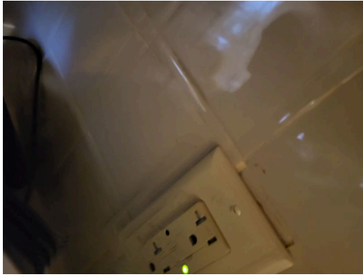
Apartment 52-3 kitchen GFCI
