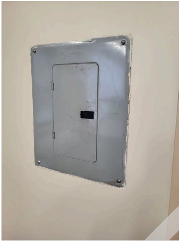
81. Gould electrical Panel
