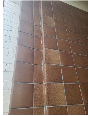
22. Building ingress/egress ceramic tile wall damage (Non-Critical Repair)
