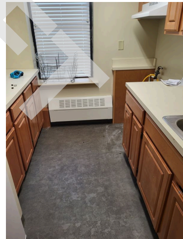
84. Community room kitchen area flooring, cabinets, countertops, range hood and hydronic baseboard
