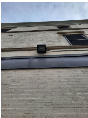
Exterior wall mounted high density light fixture
