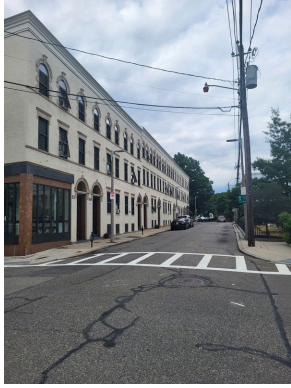
Pole electric transformer
