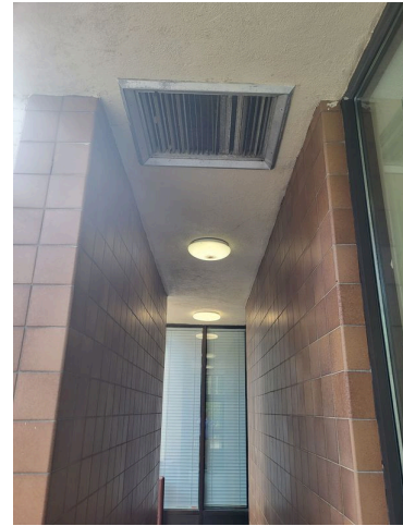
26. Common hallway light fixture
