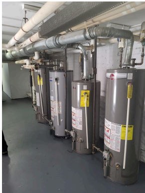
Hot water heater copper pipes
