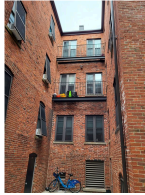
Northeast elevation court yard brick façade, balcony railings, window screens and high density light fixture
