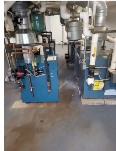
110. Boilers with copper pipes
