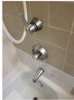
Apartment 54-2 bathroom bathtub hardware
