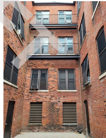
60. Southeast elevation courtyard brick façade, balcony railings, window screens and high density light fixture
