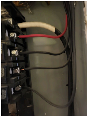
Apartment 58-3 circuit breaker box, copper lines
