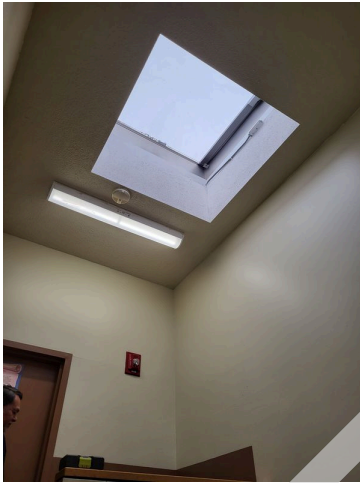
1. Common area skylight, smoke detector, emergency strobe light, and light fixture
