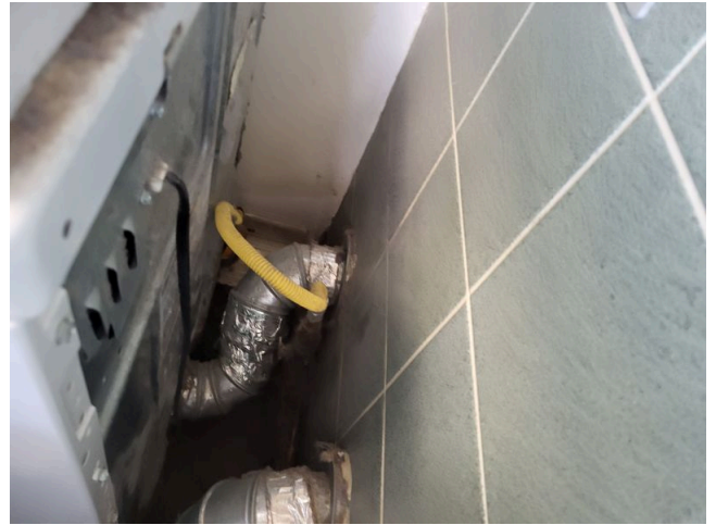
94. Laundry room dryer vent damaged (Non-Critical Repair)
