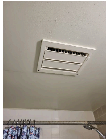
14. Apartment 54-2 bathroom ventilation
