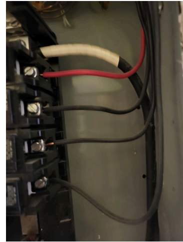
74. Apartment 58-3 circuit breaker box, copper lines
