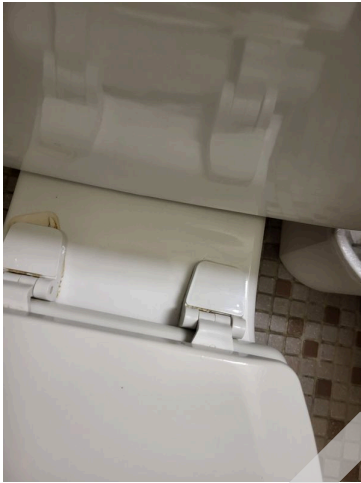
21. Apartment 54-2 bathroom toilet tank GPF
