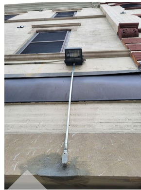
Exterior wall mounted high density light fixture
