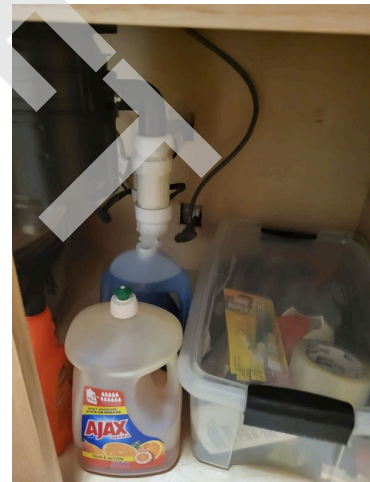
8. Apartment 54-2 kitchen garbage disposal
