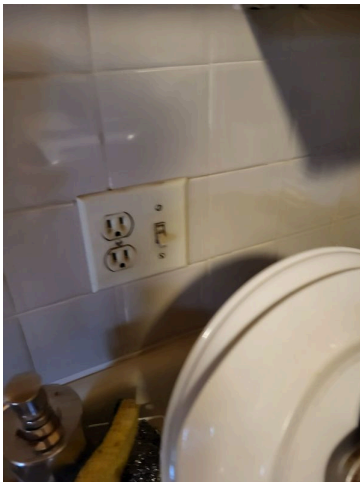
83. Apartment 52-3 kitchen outlet and switch
