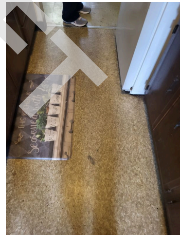
32. Apartment 56-3 kitchen sheet vinyl flooring (Non-Critical Repair)
