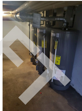
Hot water heaters
