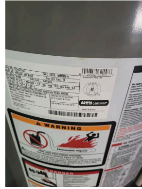
Laundry room 50 gallon hot water heater
