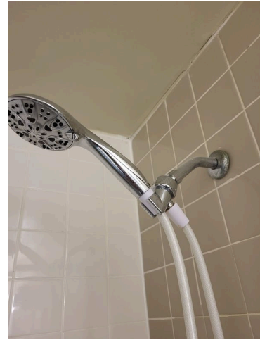
22. Apartment 54-2 bathroom shower head
