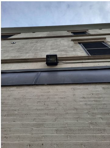
51. Exterior wall mounted high density light fixture
