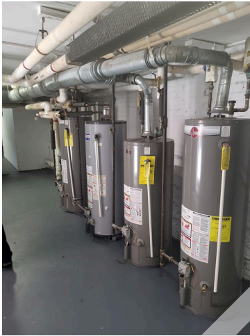
101. Hot water heater copper pipes
