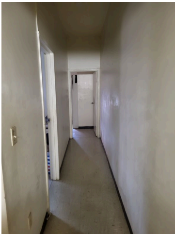
47. Apartment 56-3 hallway vinyl tile flooring (Non-Critical Repair)
