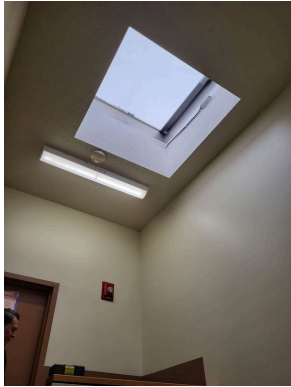
Common area stairwell sky light, light fixture and smoke detector
