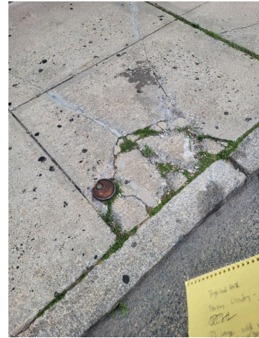
38. West elevation sidewalk damage trip hazard (Critical Repair)
