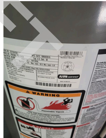
104. Laundry room 50 gallon hot water heater
