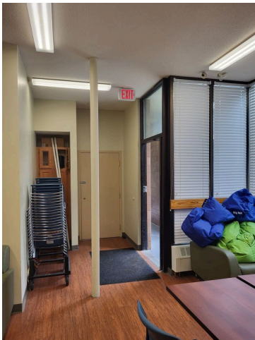
79. Community room and kitchen area emergency exit sign and emergency lighting
