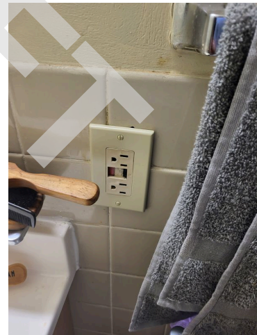
40. Apartment 56-3 bathroom GFCI
