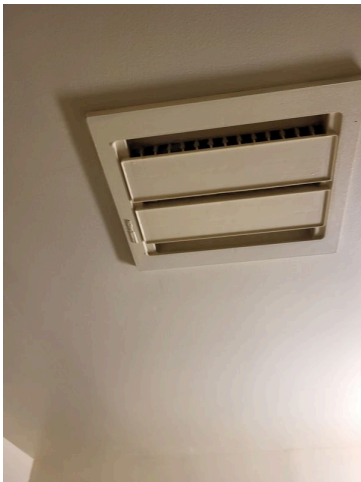
95. Apartment 52-3 bathroom ventilation
