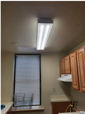
83. Community room kitchen area light fixture
