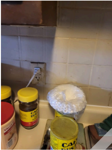
33. Apartment 56-3 kitchen GFCI
