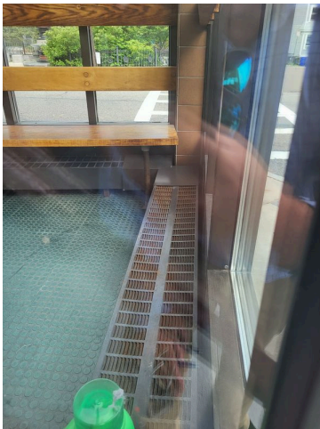
31. Common area hydronic baseboard
