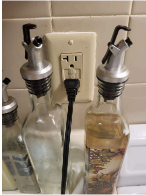
Apartment 54-2 kitchen GFCI
