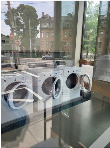
29. Common area laundry room front end loader washers
