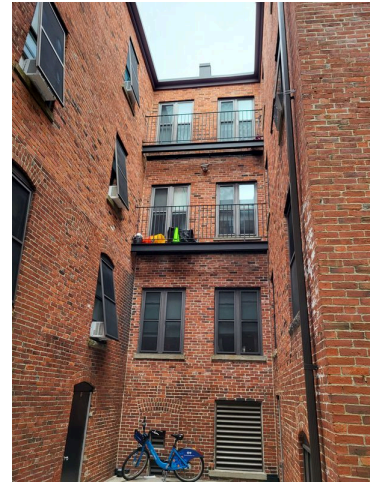
70. Northeast elevation court yard brick façade, balcony railings, window screens and high density light fixture
