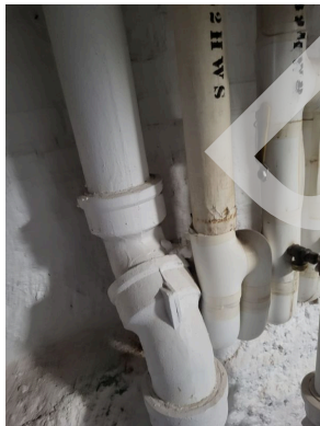
Cast iron pipe
