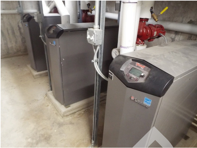
149. Heating hot water boilers - building 15
