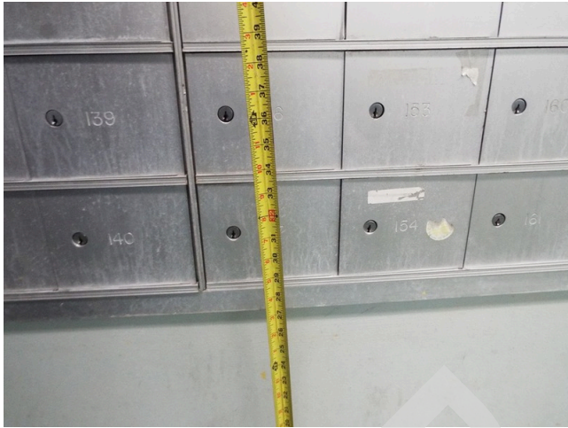
205. Common area - building 12 - mailboxes
