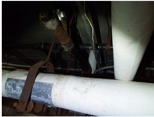
Pipe leak at repair - building 17 basement (Non-Critical Repair)
