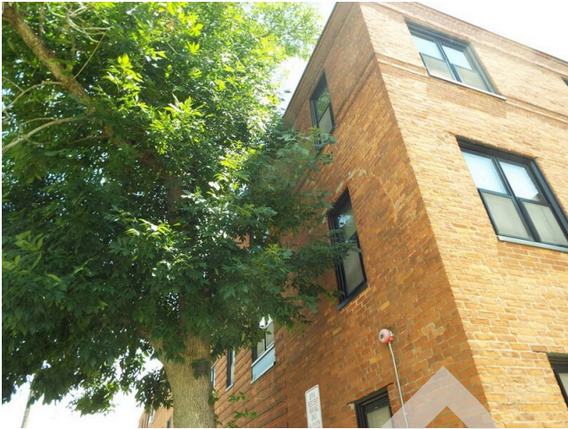
53. Overhanging tree - building 8 (Non-Critical Repair)
