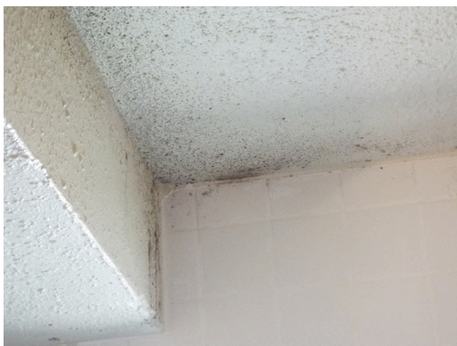
5-bed-2-bath-TH - unit 140A - building 16 - bathroom ceiling mold (Critical Repair)
