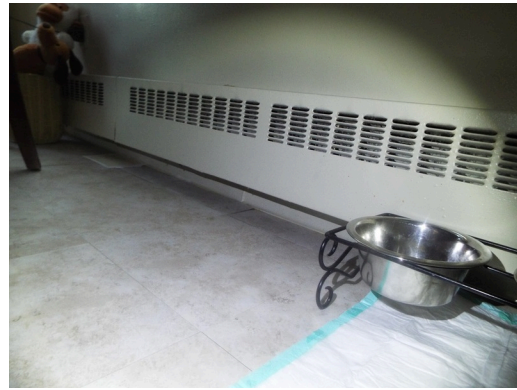
2-bed-1-bath - unit 160C - building 15 - baseboard heating unit
