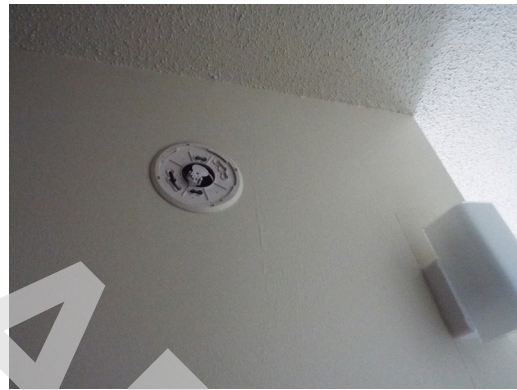
3-bed-1.5-bath-TH - unit 214 - building 3 - missing smoke detector (Critical Repair)
