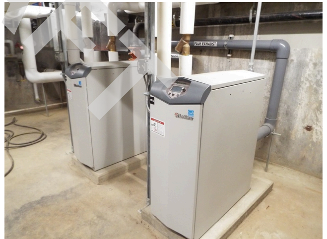
136. Domestic hot water boilers - building 15
