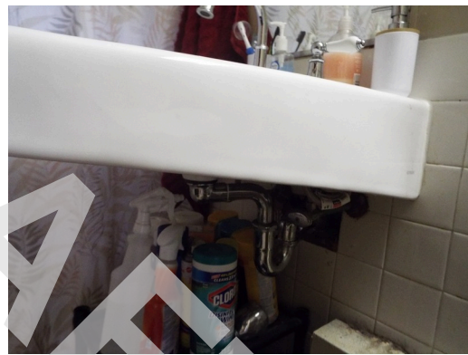
UFAS bathroom sink lacks pipe protection - unit 13 - building 4 (Critical Repair)
