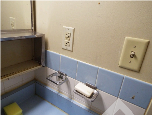
37. 1-bed-1-bath - unit 90D - building 19 - typical bathroom GFCI
