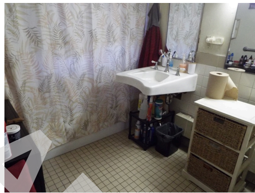
UFAS bathroom fixtures- unit 13 - building 4
