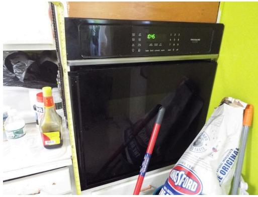
UFAS wall oven - unit 53 - building 8
