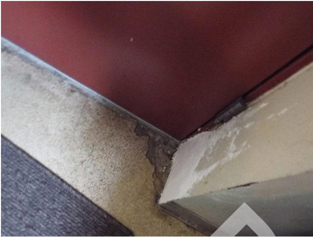
273. 3-bed-1-bath-UFAS - unit 13 - building 4 - wall condition (Non-Critical Repair)
