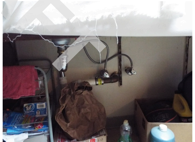
236. UFAS kitchen sink lacks pipe protection - unit 13 - building 4
