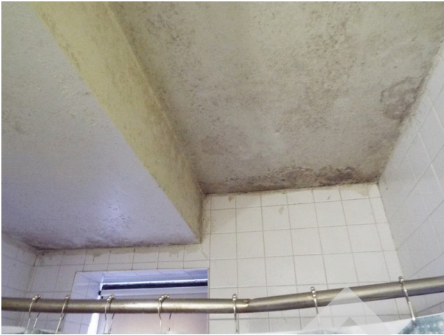
345. 3-bed-1.5 bath - unit 42 - building 17 - bathroom ceiling mold (Critical Repair)
