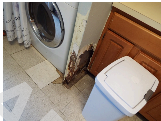
3-bed-1.5-bath-TH - unit 22 - building 17 - washer wall condition (Non-Critical Repair)
