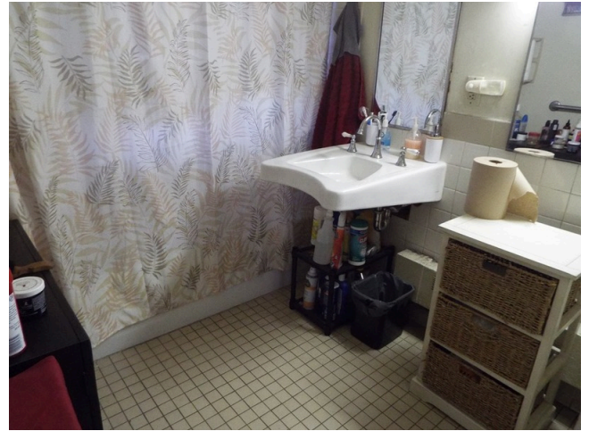
246. UFAS bathroom fixtures- unit 13 - building 4
