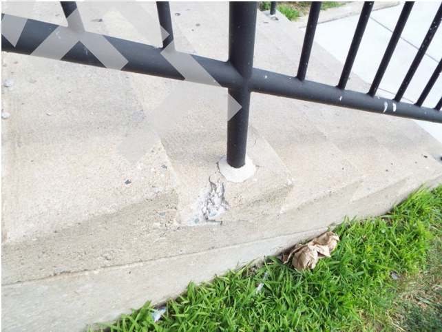
40. Concrete step spalling - building 17 (Non-Critical Repair)
