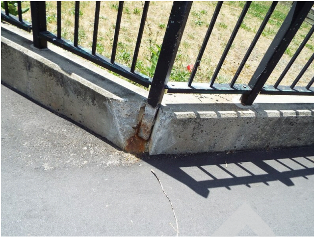
9. Concrete retaining wall spalling - rear building 9 (Non-Critical Repair)
