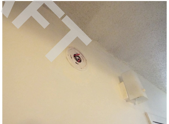
344. 2-bed-1-bath - unit 82 - building 7 UFAS - missing smoke detector (Critical Repair)
