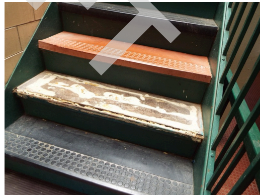
Interior stair tread condition - building 7 (Critical Repair)
