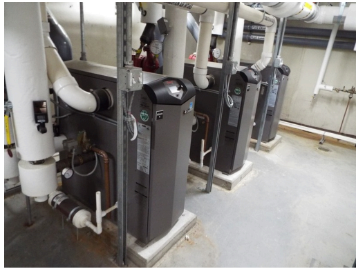
Heating hot water boilers - building 18
