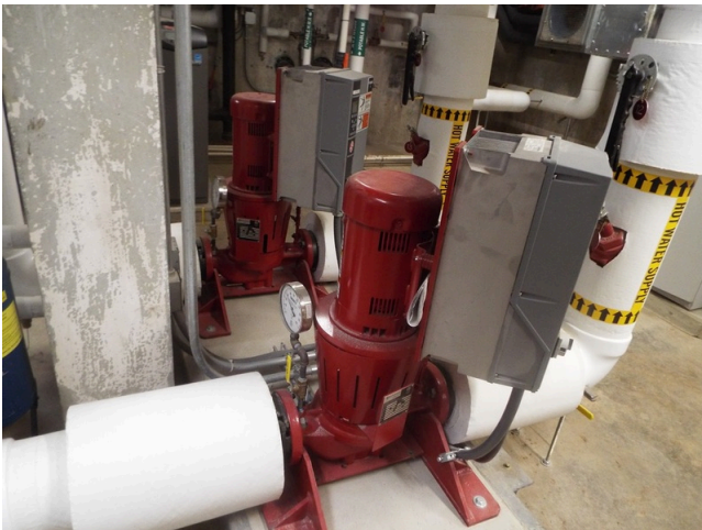
151. Heating hot water pumps - building 15
