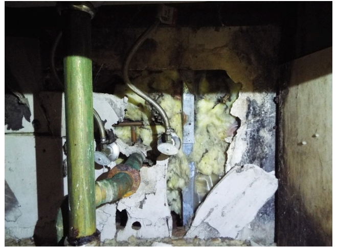
354. 4-bed-2-bath - unit 17 - building 4 wall damage (Non-Critical Repair)
