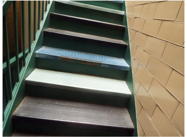
186. Interior stair tread condition - building 15 (Critical Repair)
