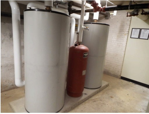
Domestic hot water storage tanks - building 15
