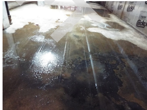
Moisture at pipe leak - building 17 basement (Non-Critical Repair)
