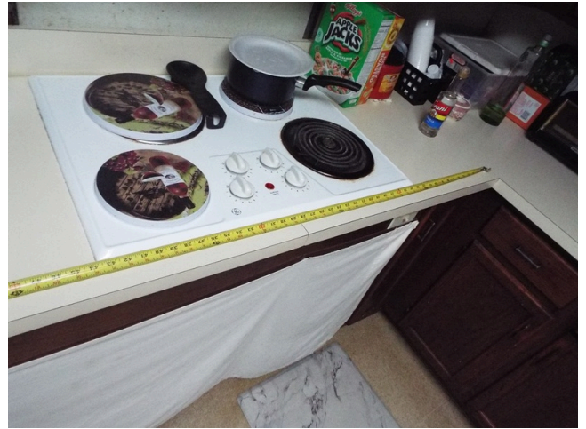
238. UFAS cooktop - unit 13 - building 4
