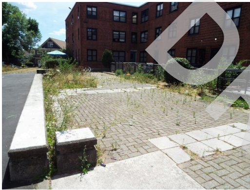
Overgrown vegetation - building 7 (Non-Critical Repair)
