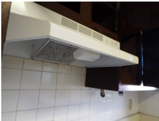
1-bed-1-bath - unit 90D - building 19 - range hood
