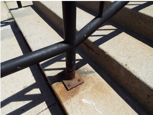
43. Handrail post base condition - building 12 (Non-Critical Repair)
