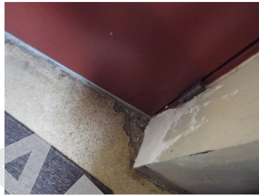
3-bed-1-bath-UFAS - unit 13 - building 4 - wall condition (Non-Critical Repair)
