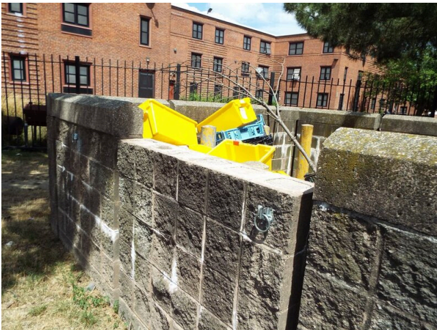
67. Missing dumpster enclosure cap section - building 1 (Non-Critical Repair)
