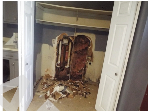
4-bed-2-bath-TH - unit 218 - building 3 - laundry wall condition (Non-Critical Repair)
