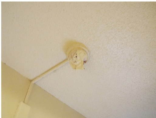
5-bed-2-bath-TH - unit 190A - building 14 - disabled smoke detector (Critical Repair)
