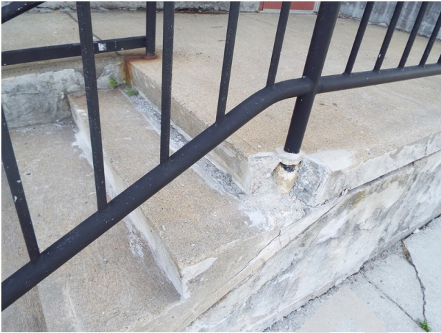
41. Concrete step spalling - building 19 (Non-Critical Repair)
