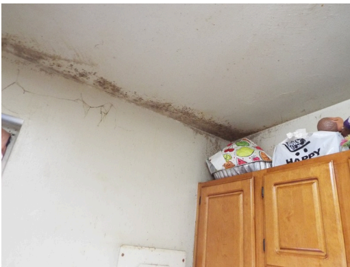
1-bed-1-bath - unit 21A - building 6 - kitchen ceiling mold (Critical Repair)
