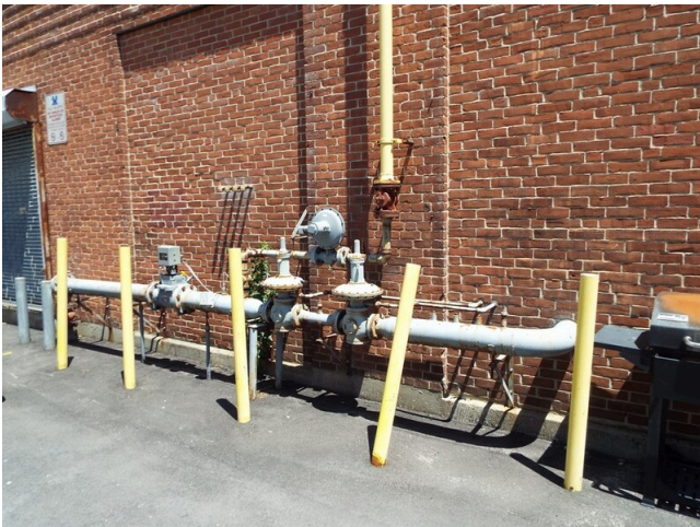
75. Gas meter - building 12
