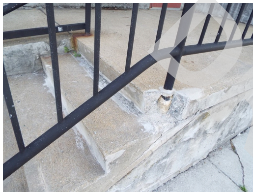
Concrete step spalling - building 19 (Non-Critical Repair)
