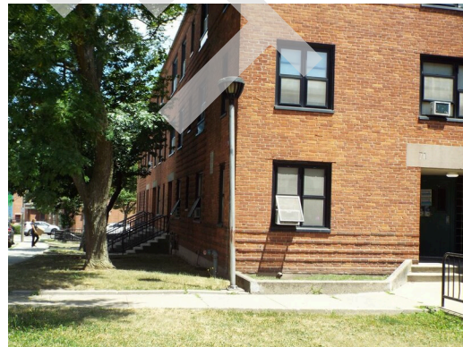
Decorative pole mounted lighting condition (Non-Critical Repair)
