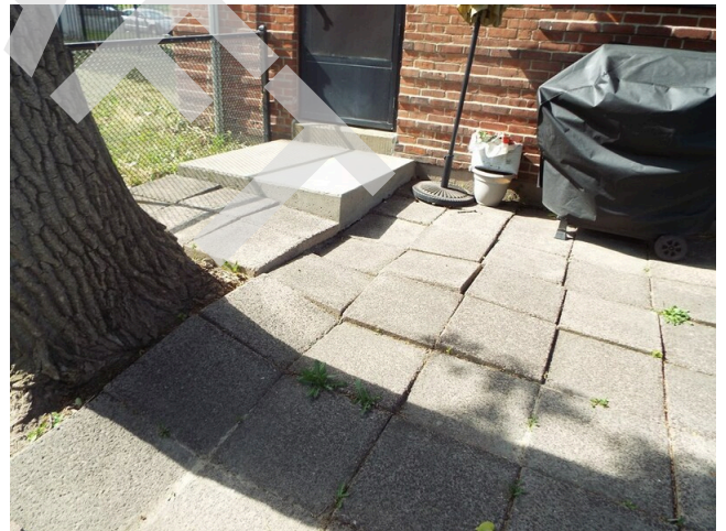
84. Concrete patio paver condition - building 15 (Critical Repair)
