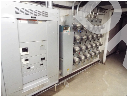
Main electrical distribution panel and meters - building 18
