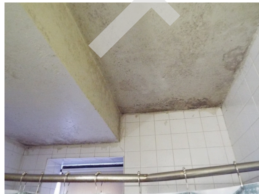
3-bed-1.5 bath - unit 42 - building 17 - bathroom ceiling mold (Critical Repair)
