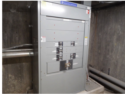
Main electric distribution panel - building 15
