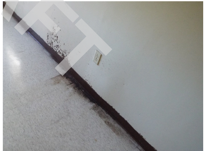
152. 3-bed-1.5-bath-TH - unit 160B - building 13 - wall mold (Critical Repair)
