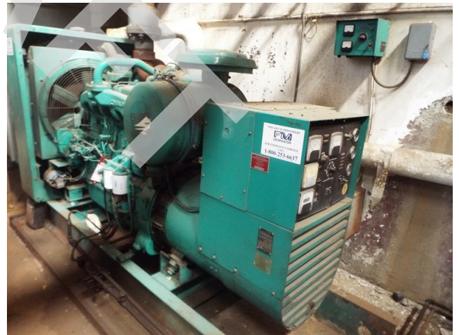
156. Emergency generator - building 12
