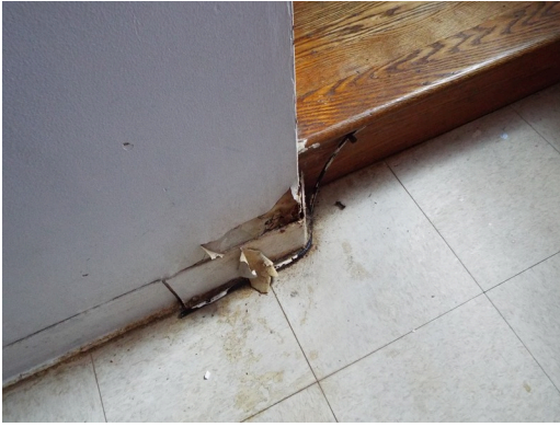
4-bed-2-bath - unit 17 - building 4 - wall condition (Non-Critical Repair)
