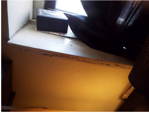
3-bed-1-bath-UFAS - unit 13 - building 4 - termites reported (Non-Critical Repair)
