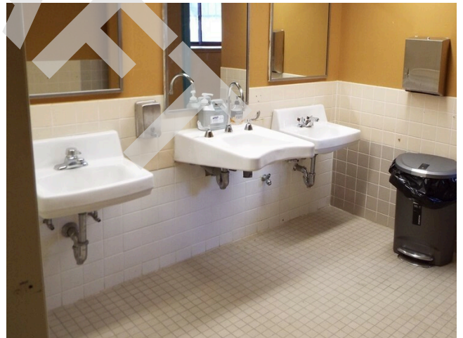
188. Common area - building 18 - teen center - women's restroom 2 of 3 sinks lack pipe protection (Critical Repair)
