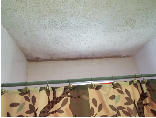
2-bed-1-bath - unit 230D - building 1 - bathroom ceiling mold (Critical Repair)
