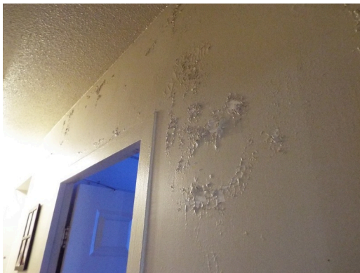
2-bed-1-bath - unit 50E - building 18 - wall paint condition (Non-Critical repair)
