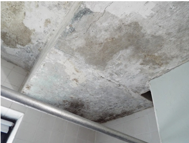
119. 3-bed-1.5-bath-TH - unit 22 - building 17 - bathroom ceiling condition (Critical Repair)
