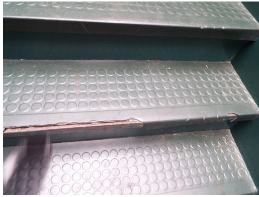
Interior stair tread condition - building 19 (Critical Repair)
