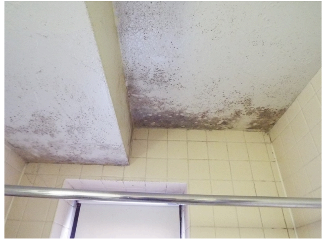
362. 1-bed-1-bath - unit 21A - building 6 - bathroom ceiling mold (Critical Repair)
