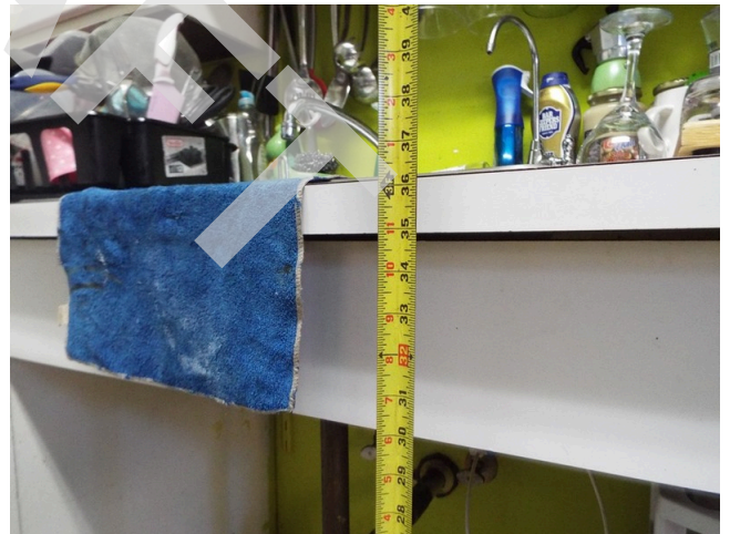
180. 4-bed-2-bath-UFAS - unit 53 - building 8, too high (Critical Repair)
