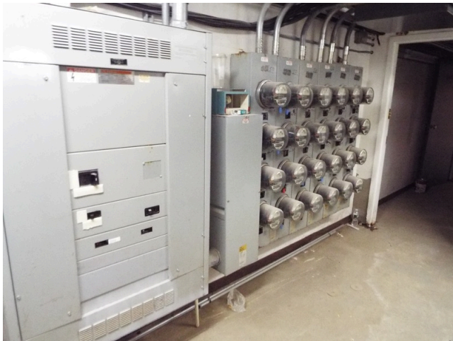
155. Main electrical distribution panel and meters - building 18
