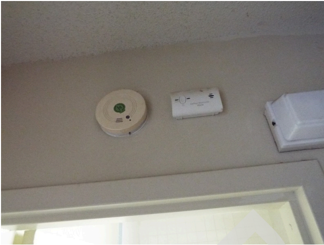
25. 1-bed-1-bath - unit 90D - building 19 - hall smoke and CO2 detectors
