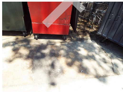
Dumpster pad condition - building 10 (Non-Critical Repair)
