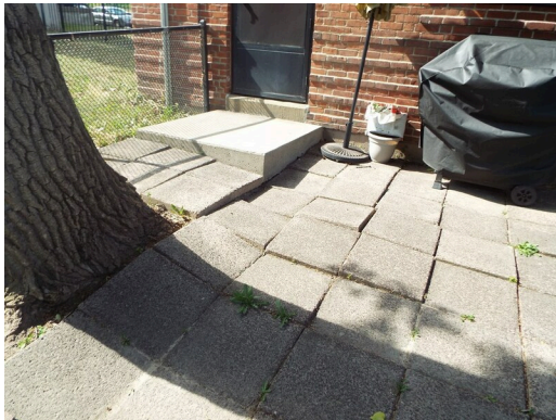
Concrete patio paver condition - building 15 (Critical Repair)
