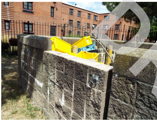
Missing dumpster enclosure cap section - building 1 (Non-Critical Repair)
