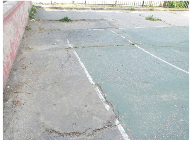
74. Basketball court surface condition (Non-Critical Repair)
