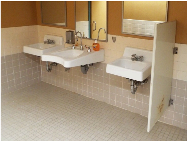
187. Common area - building 18 - teen center - men's restroom 2 of 3 sinks lack pipe protection (Critical Repair)
