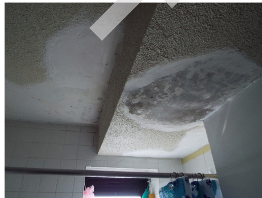
4-bed-2-bath - unit 17 - building 4 - bathroom ceiling mold (Critical Repair)
