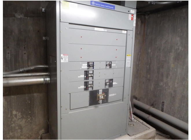
154. Main electric distribution panel - building 15
