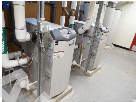
Domestic hot water boilers - building 18
