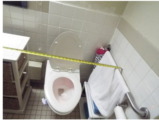
UFAS toilet lacks rear grab bar- unit 13 - building 4 (Critical Repair)
