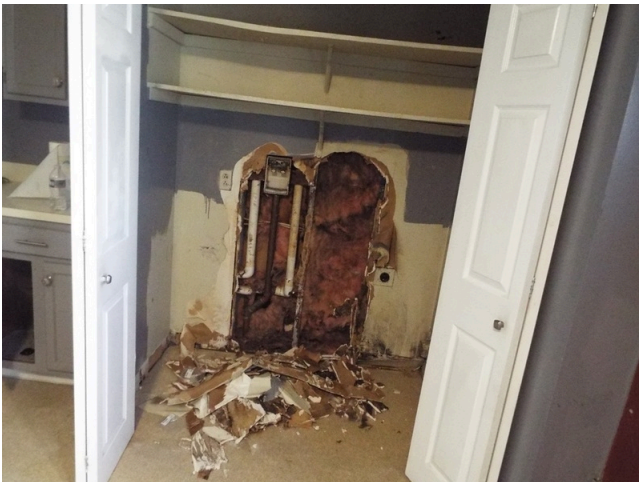
295. 4-bed-2-bath-TH - unit 218 - building 3 - laundry wall condition (Non-Critical Repair)
