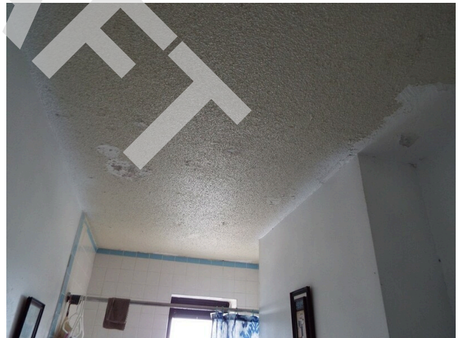
360. 4-bed-2-bath - unit 17 - building 4 - ceiling condition (Non-Critical Repair)
