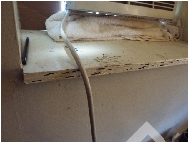
265. 3-bed-1-bath-UFAS - unit 13 - building 4 - termites reported (Non-Critical Repair)
