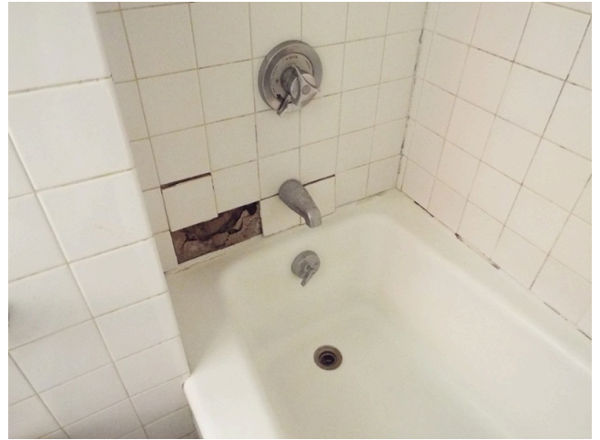
346. 3-bed-1.5 bath - unit 42 - building 17 - bathroom shower tile condition (Non-Critical Repair)
