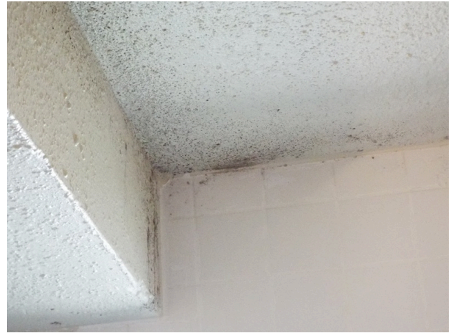
322. 5-bed-2-bath-TH - unit 140A - building 16 - bathroom ceiling mold (Critical Repair)
