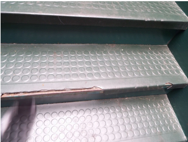
183. Interior stair tread condition - building 19 (Critical Repair)
