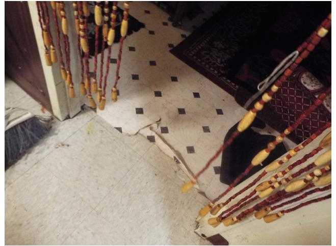
314. 5-bed-2-bath-TH - unit 140A - building 16 - flooring condition (Non-Critical Repair)
