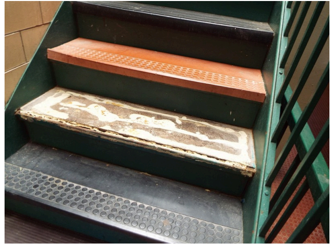
182. Interior stair tread condition - building 7 (Critical Repair)
