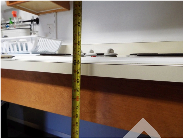
365. UFAS unit 172 - building 13 - kitchen sink counters exceed 34 inch height (Critical Repair)
