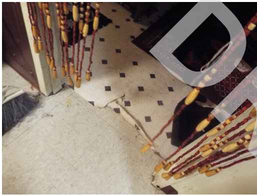
5-bed-2-bath-TH - unit 140A - building 16 - flooring condition (Non-Critical Repair)
