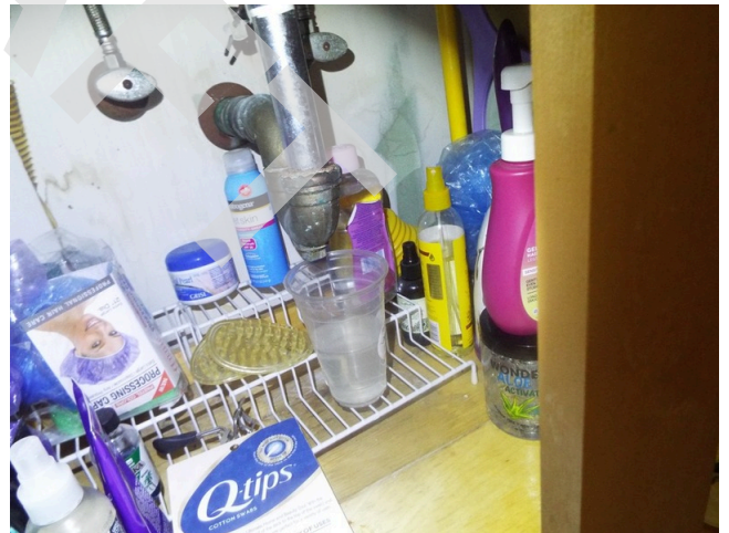
80. 2-bed-1-bath - unit 160C - building 15 - rodents reported - kitchen (Critical Repair)
