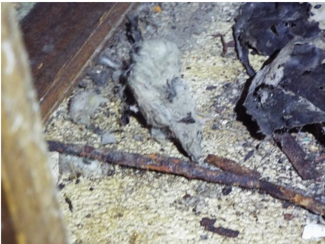
355. 4-bed-2-bath - unit 17 - building 4 - dead rodent (Critical Repair)
