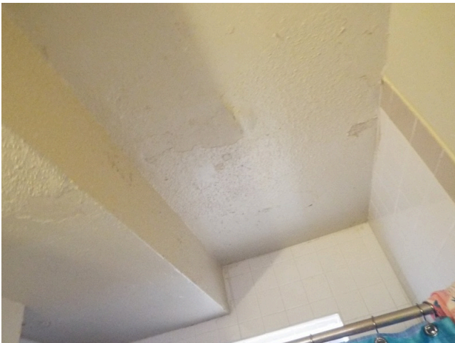
331. 5-bed-2-bath-TH - unit 190A - building 14 - bathroom paint condition (Non-Critical Repair)
