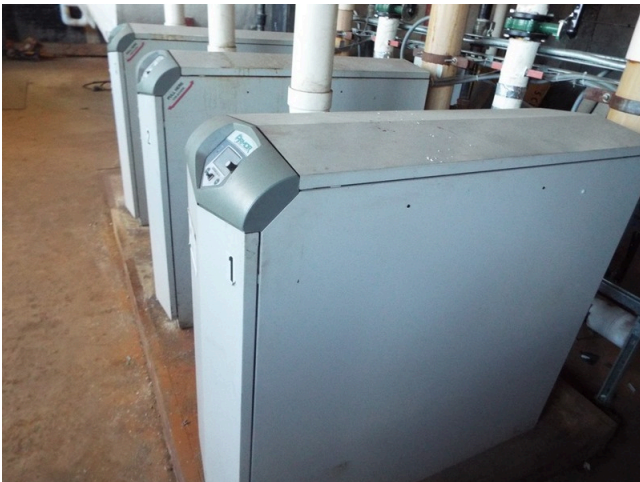
135. Domestic hot water boilers - building 12
