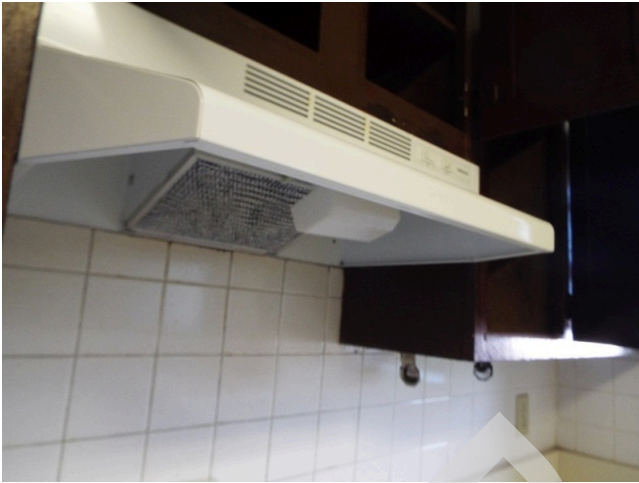
13. 1-bed-1-bath - unit 90D - building 19 - range hood
