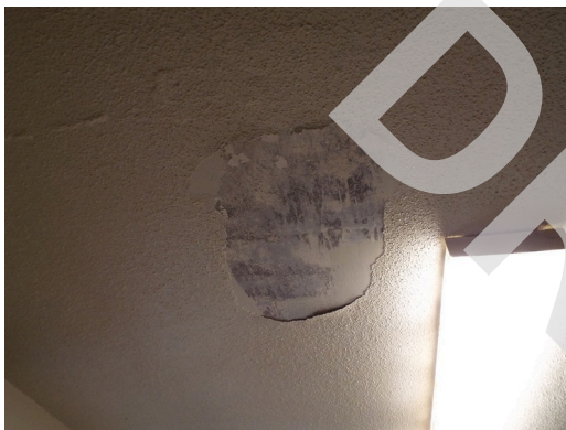
2-bed-1-bath - unit 240A - building 1 - ceiling paint condition (Non-Critical Repair)
