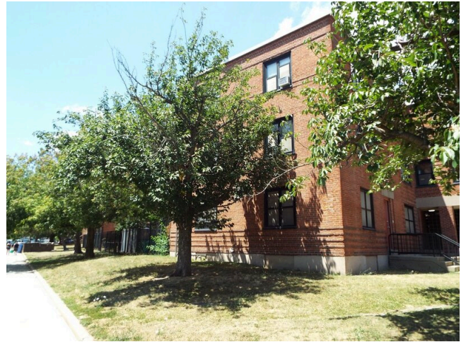
54. Overhanging tree - building 12 (Non-Critical Repair)
