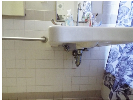
UFAS bathroom sink lacks pipe protection - unit 53 - building 8 (Critical Repair)
