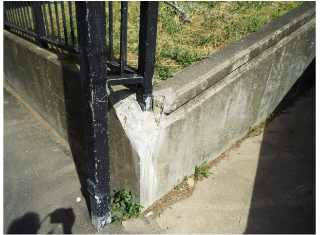
6. Concrete retaining wall spalling - building 19 (Non-Critical Repair)
