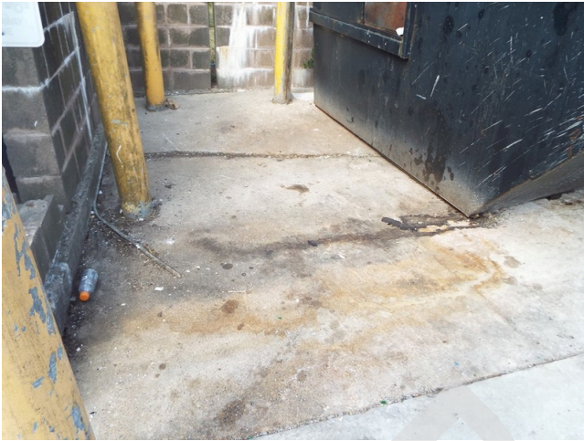
29. Dumpster pad condition - building 14-17 (Non-Critical Repair)
