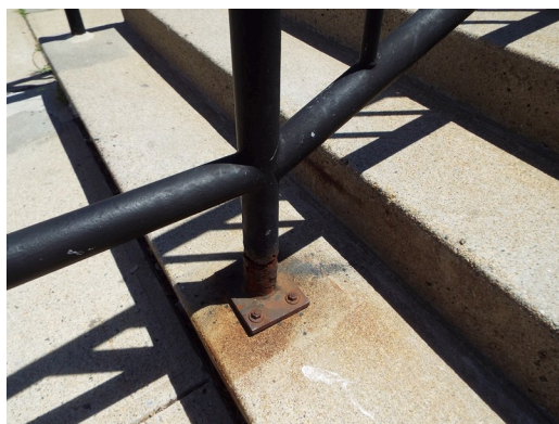
Handrail post base condition - building 12 (Non-Critical Repair)
