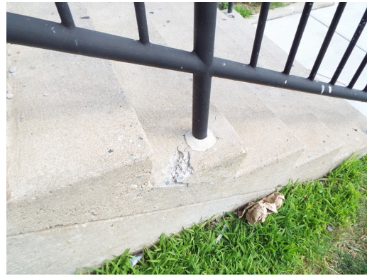
Concrete step spalling - building 17 (Non-Critical Repair)
