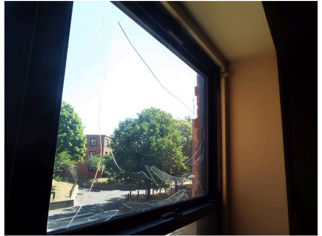
50. 2-bed-1-bath - unit 100B - building 12 - broken window glass (Critical Repair)
