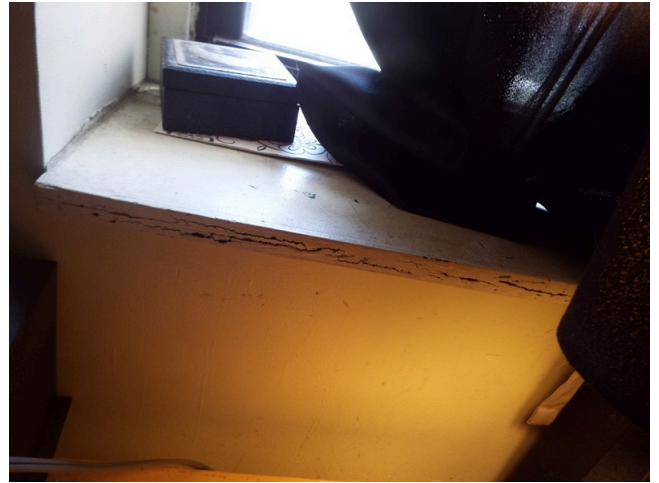
266. 3-bed-1-bath-UFAS - unit 13 - building 4 - termites reported (Non-Critical Repair)
