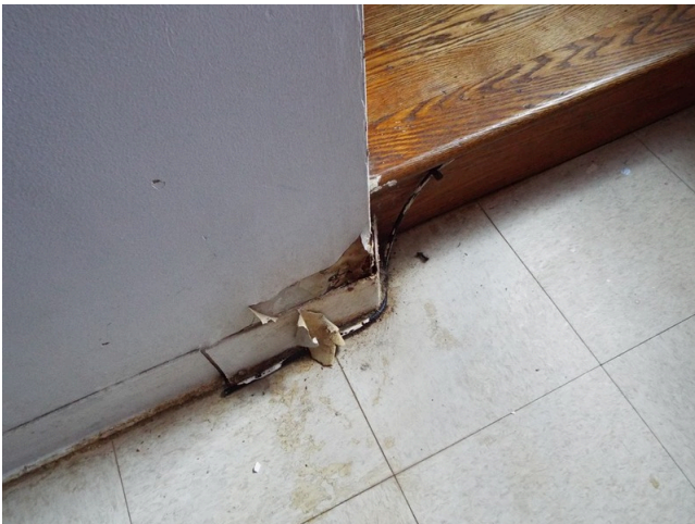
359. 4-bed-2-bath - unit 17 - building 4 - wall condition (Non-Critical Repair)
