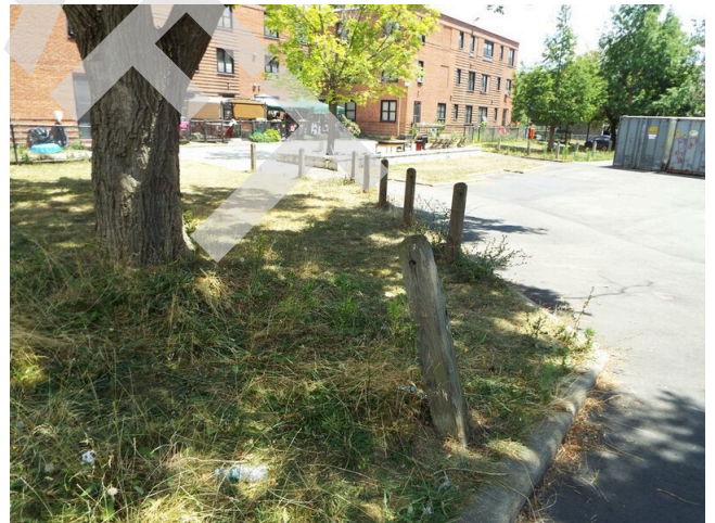
60. Wood fence post condition - rear buildings 9-12(Non-Critical Repair)
