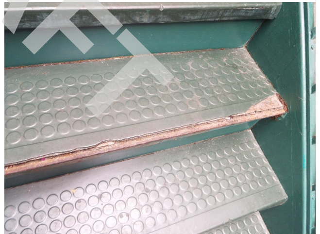
184. Interior stair tread condition - building 19 (Critical Repair)
