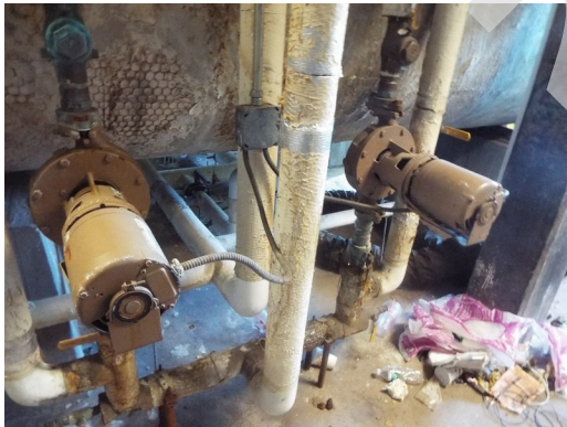
Domestic hot water circulation pumps - building 12
