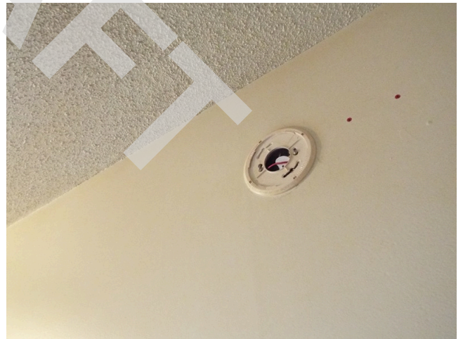
340. 1-bed-1-bath - unit 31E - building 6 - missing smoke detector (Critical Repair)
