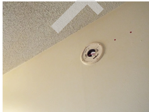
1-bed-1-bath - unit 31E - building 6 - missing smoke detector (Critical Repair)
