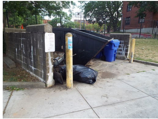
Missing dumpster enclosure cap section - building 15-16 (Non-Critical Repair)
