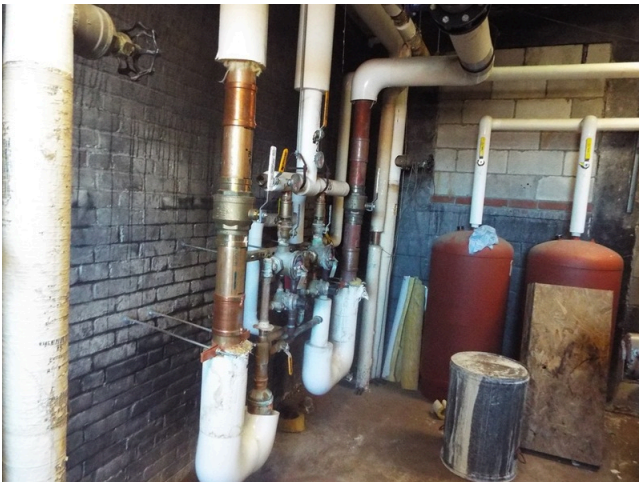
147. Domestic hot water mixing valves - building 12
