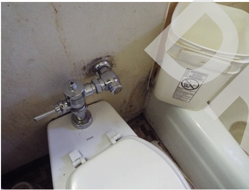
1-bed-1-bath - unit 21A - building 6 - bathroom wall condition (Non-Critical Repair)
