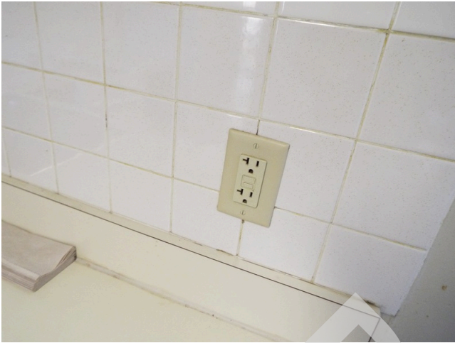
9. 1-bed-1-bath - unit 90D - building 19 - typical kitchen GFCI
