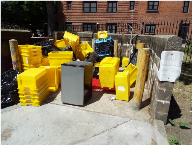
25. Dumpster pad condition - building 1 (Non-Critical Repair)
