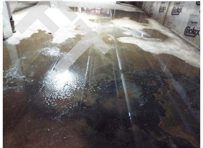
144. Moisture at pipe leak - building 17 basement (Non-Critical Repair)
