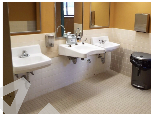
Common area - building 18 - teen center - women's restroom 2 of 3 sinks lack pipe protection (Critical Repair)
