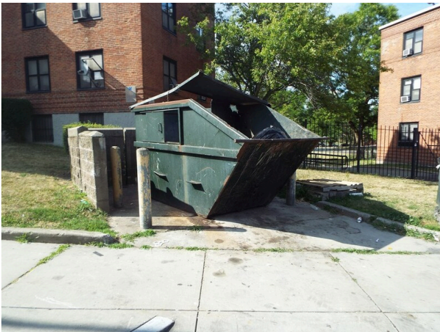
31. Dumpster pad condition - building 18-19 (Non-Critical Repair)
