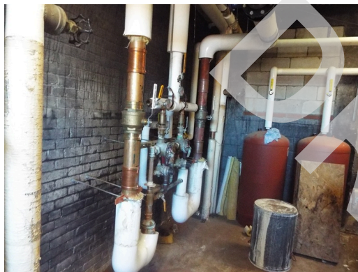
Domestic hot water mixing valves - building 12
