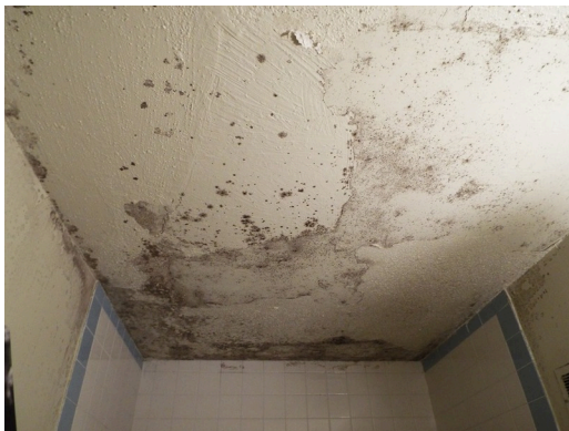
3-bed-1.5-bath-TH - unit 214 - building 3 - bathroom ceiling mold (Critical Repair)
