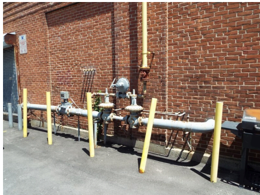
Gas meter - building 12
