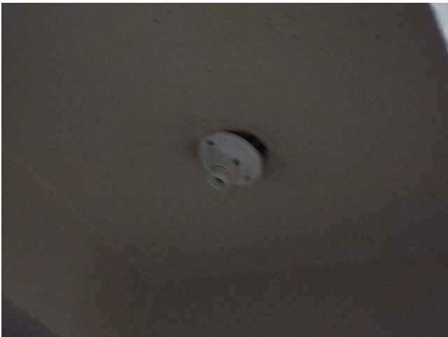
343. 2-bed-1-bath - unit 50G - building 18 - loose light fixture (Critical Repair)
