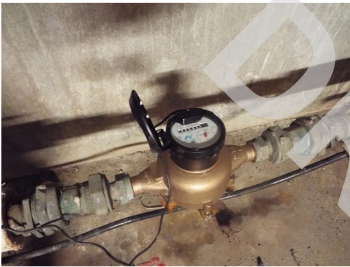
Water meter - building 15
