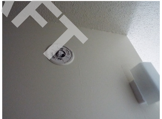
168. 3-bed-1.5-bath-TH - unit 214 - building 3 - missing smoke detector (Critical Repair)
