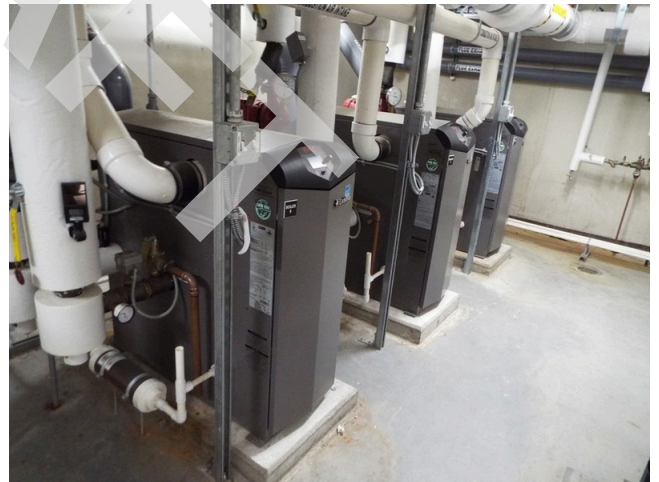
152. Heating hot water boilers - building 18
