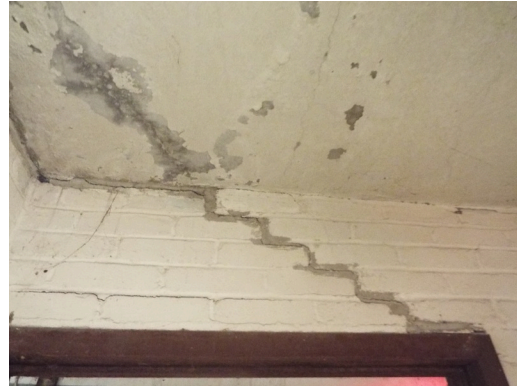
Masonry wall cracks - basement building 15 (Non-Critical Repair)
