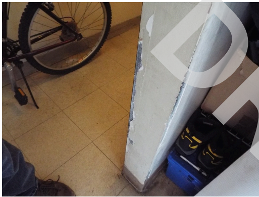
3-bed-1-bath-UFAS - unit 13 - building 4 - wall condition (Non-Critical Repair)
