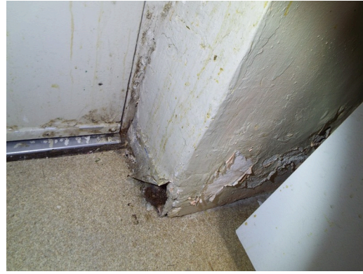
3-bed-1.5 bath - unit 42 - building 17 - bathroom wall condition (Non-Critical Repair)
