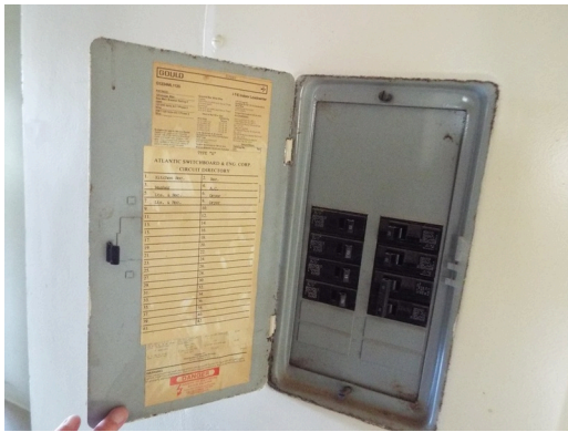
1-bed-1-bath - unit 90D - building 19 - unit electrical panel
