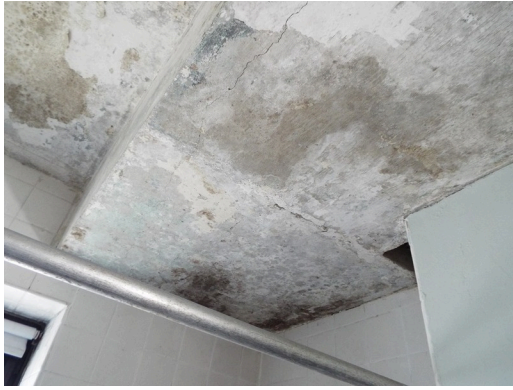
3-bed-1.5-bath-TH - unit 22 - building 17 - bathroom ceiling condition (Critical Repair)
