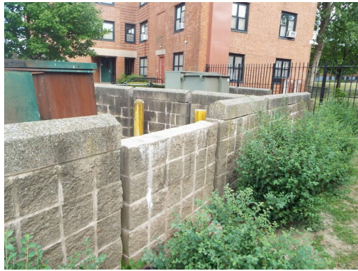
Missing dumpster enclosure cap section - building 14-15 (Non-Critical Repair)
