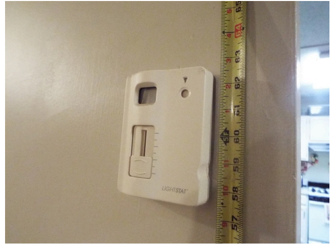
366. UFAS thermostat exceeds 54 inch height - unit 38 building 2 (Critical Repair)
