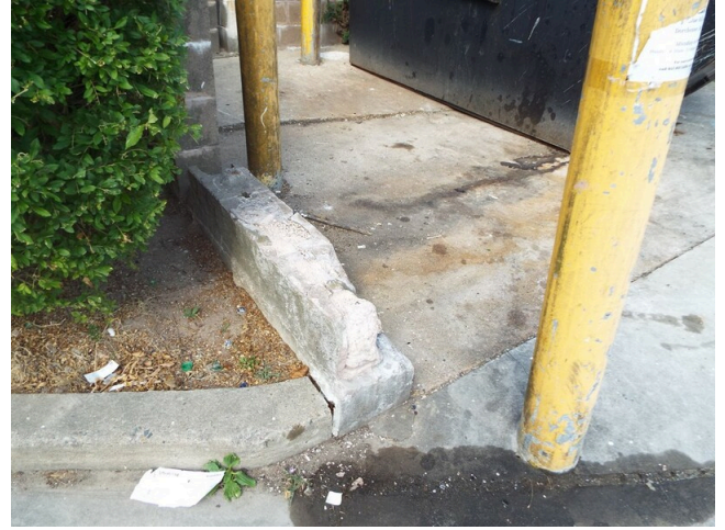
66. Dumpster wall damage - building 14-17 (Non-Critical Repair)
