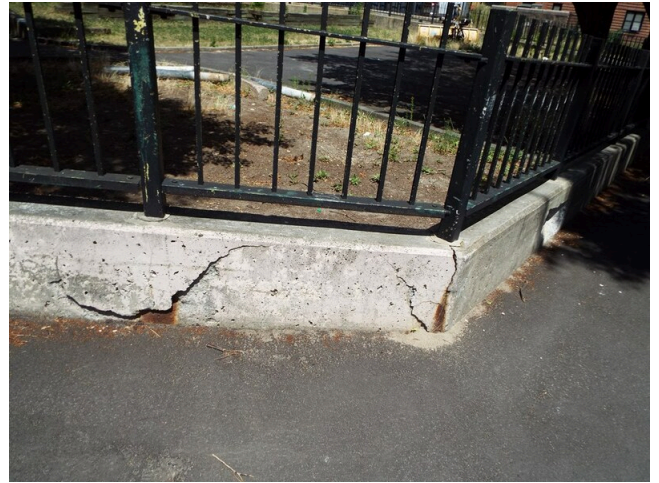
10. Concrete retaining wall spalling - rear building 9 (Non-Critical Repair)
