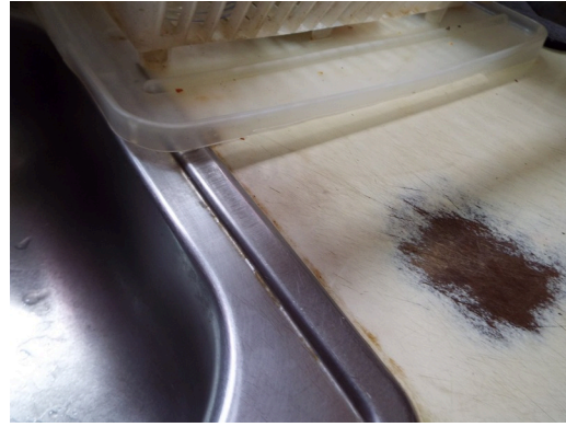
4-bed-2-bath - unit 17 - building 4 - kitchen counter wear (Non-Critical Repair)
