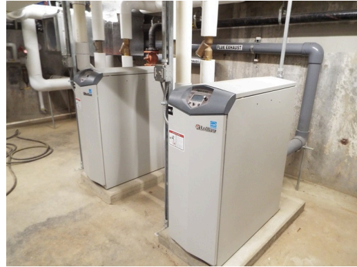
Domestic hot water boilers - building 15
