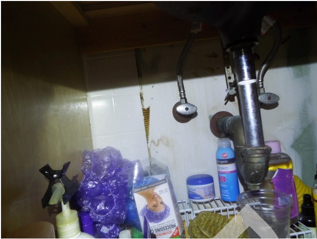
73. 2-bed-1-bath - unit 160C - building 15 - rodents reported - kitchen (Critical Repair)
