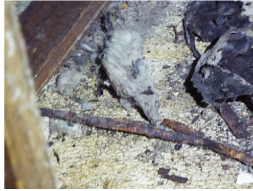
4-bed-2-bath - unit 17 - building 4 - dead rodent (Critical Repair)
