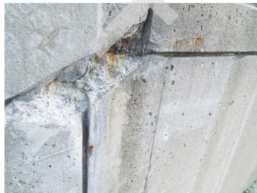
Concrete stair spalling - building 15 (Non-Critical Repair)
