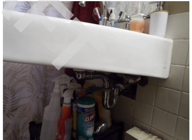
248. UFAS bathroom sink lacks pipe protection - unit 13 - building 4 (Critical Repair)
