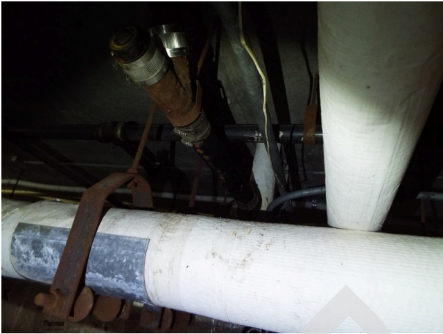
145. Pipe leak at repair - building 17 basement (Non-Critical Repair)
