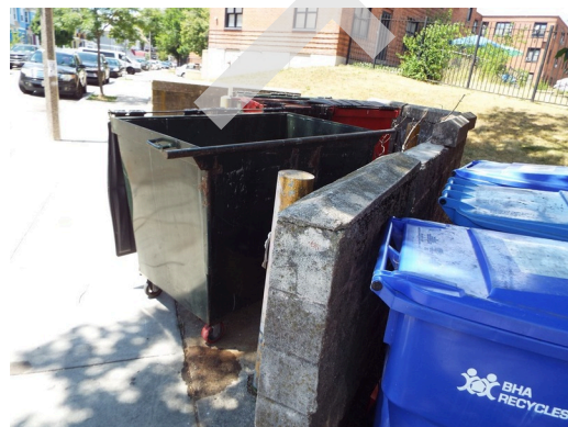
Missing dumpster enclosure cap section - building 10 (Non-Critical Repair)
