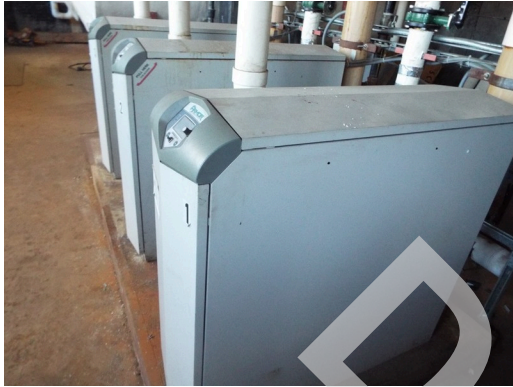
Domestic hot water boilers - building 12
