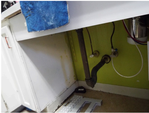
UFAS kitchen sink lacks pipe protection - unit 53 - building 8 (Critical Repair)
