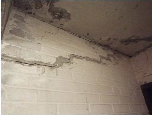
Masonry wall cracks - basement building 15 (Non-Critical Repair)
