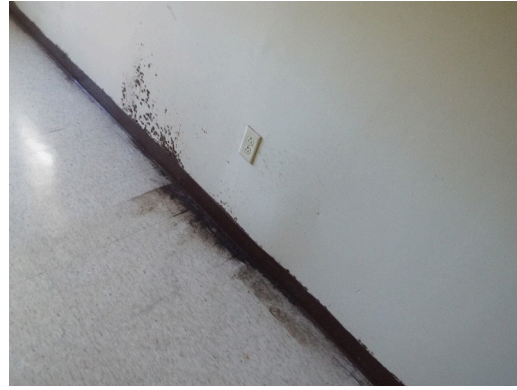
3-bed-1.5-bath-TH - unit 160B - building 13 - wall mold (Critical Repair)
