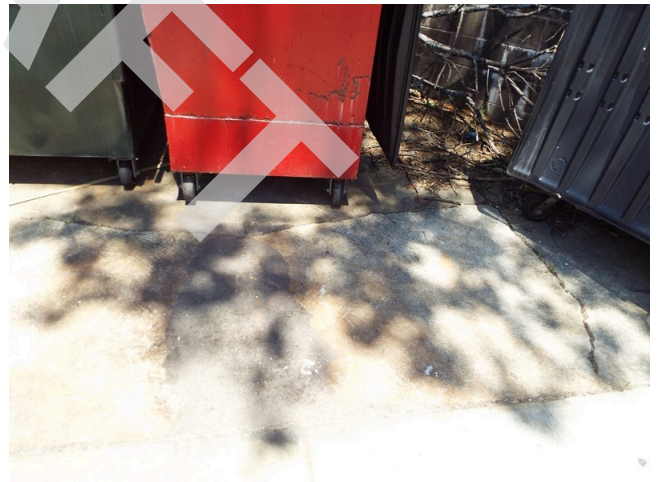
28. Dumpster pad condition - building 10 (Non-Critical Repair)
