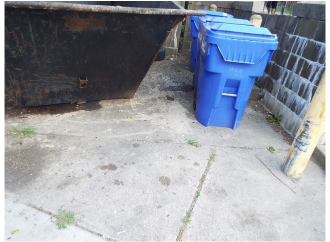
30. Dumpster pad condition - building 15-16 (Non-Critical Repair)
