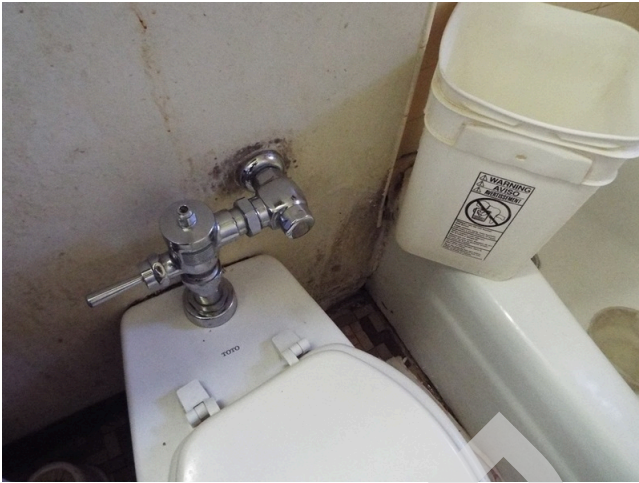
361. 1-bed-1-bath - unit 21A - building 6 - bathroom wall condition (Non-Critical Repair)
