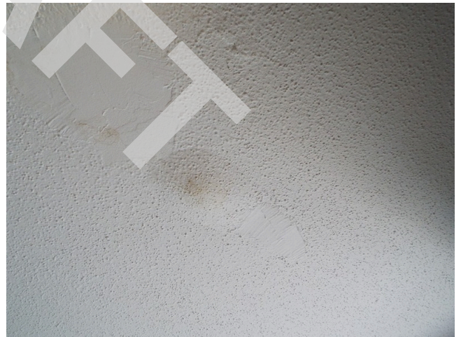
348. 3-bed-1-bath-UFAS - unit 58 - building 8 - kitchen ceiling condition (Non-Critical Repair)
