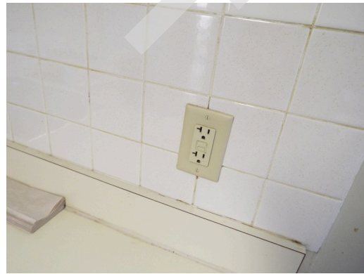
1-bed-1-bath - unit 90D - building 19 - typical kitchen GFCI
