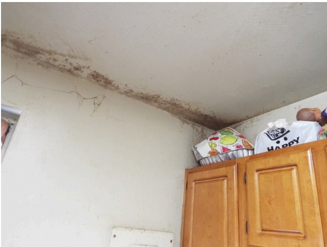
363. 1-bed-1-bath - unit 21A - building 6 - kitchen ceiling mold (Critical Repair)
