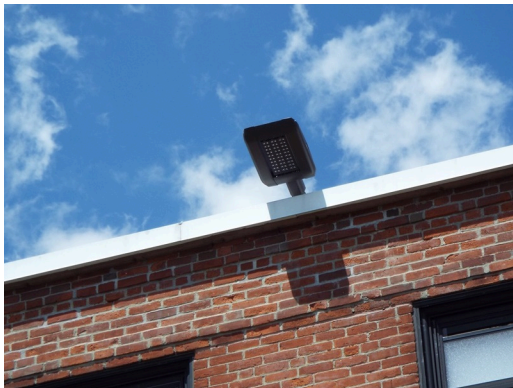
Building mounted lighting
