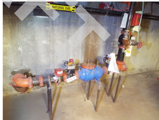
Fire sprinkler riser - building 15
