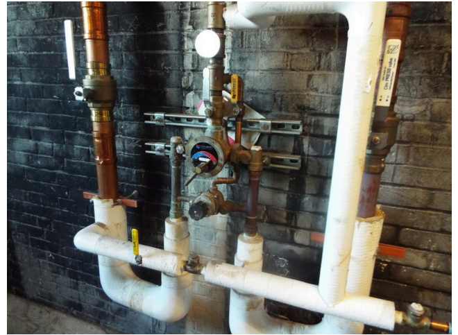
138. Domestic hot water mixing valves - building 12 (2)
