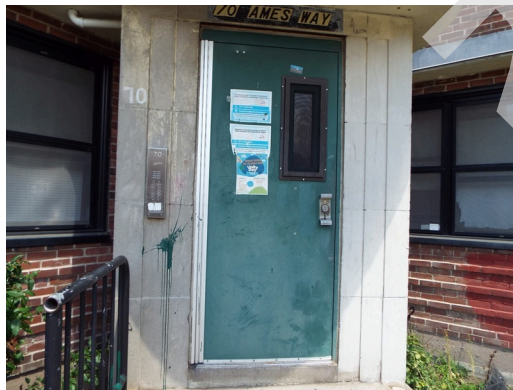
Building entry door condition - building 7 (Non-Critical Repair)
