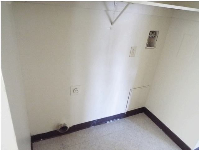
71. 2-bed-1-bath - unit 140E - building 12 - laundry hookups
