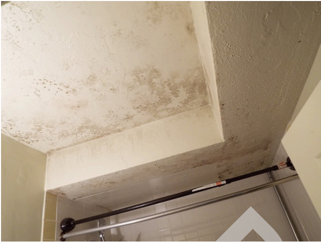
149. 3-bed-1.5-bath-TH - unit 160B - building 13 - bathroom ceiling mold (Critical Repair)
