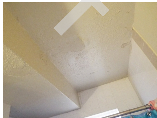
5-bed-2-bath-TH - unit 190A - building 14 - bathroom paint condition (Non-Critical Repair)
