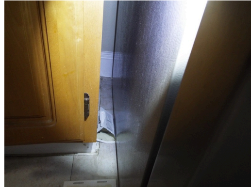
2-bed-1-bath - unit 160C - building 15 - rodents reported - kitchen (Critical Repair)
