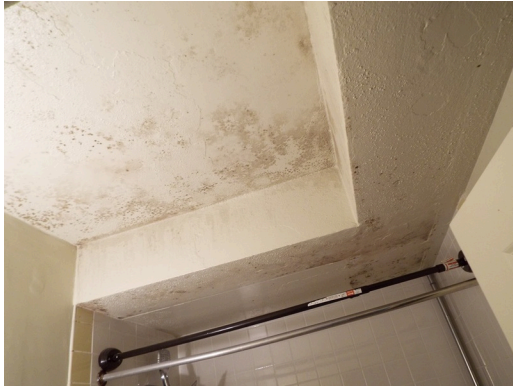
3-bed-1.5-bath-TH - unit 160B - building 13 - bathroom ceiling mold (Critical Repair)
