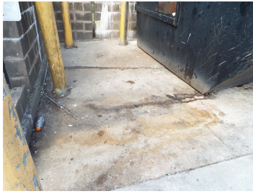
Dumpster pad condition - building 14-17 (Non-Critical Repair)
