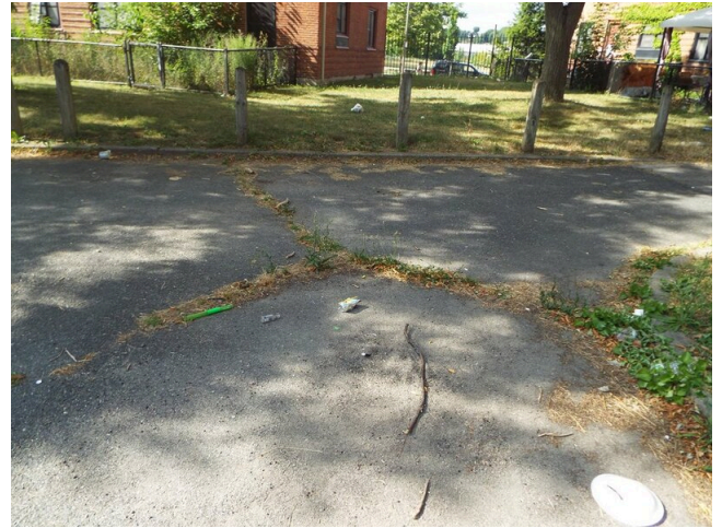
22. Asphalt pavement cracking building 3 rear (Non-Critical Repair)
