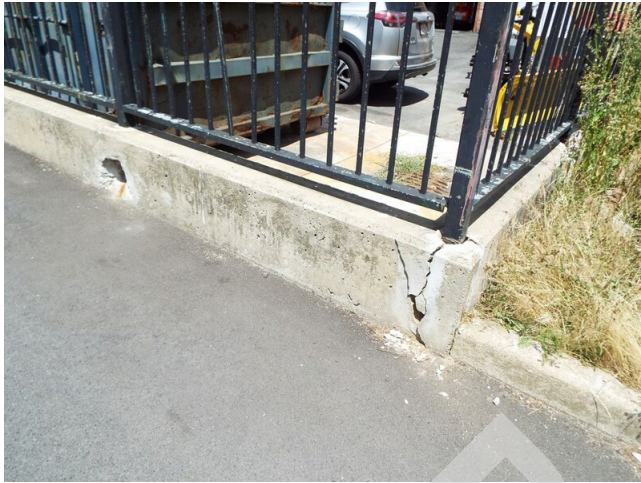
13. Concrete retaining wall spalling - rear building 12 (Non-Critical Repair)
