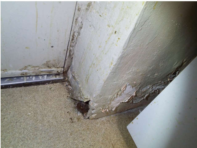
347. 3-bed-1.5 bath - unit 42 - building 17 - bathroom wall condition (Non-Critical Repair)
