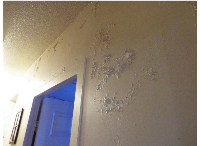
342. 2-bed-1-bath - unit 50E - building 18 - wall paint condition (Non-Critical repair)
