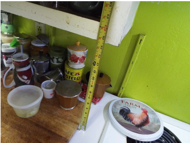
367. UFAS kitchen cabinet shelf exceeds 48 inch height - unit 13 - building 4 (Critical Repair)
