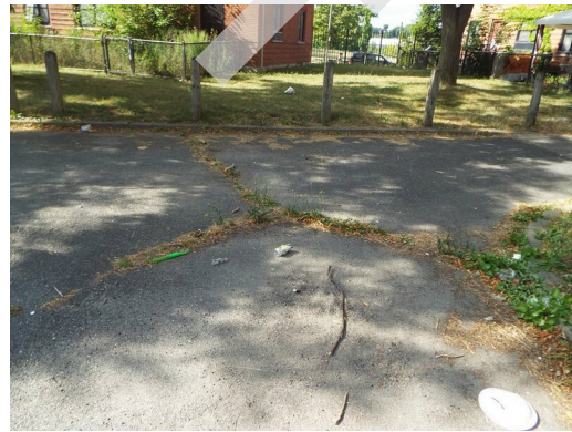
Asphalt pavement cracking building 3 rear (Non-Critical Repair)
