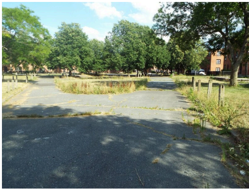
Asphalt paving - rear buildings 1 thru 6 (Non-Critical Repair)
