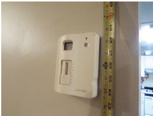
UFAS thermostat exceeds 54 inch height - unit 38 building 2 (Critical Repair)
