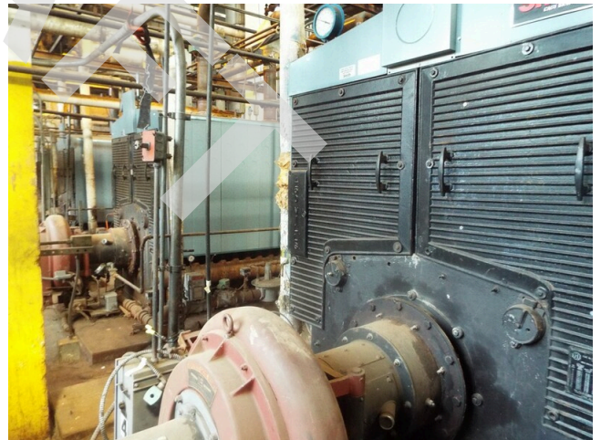
148. Heating hot water boilers - building 12
