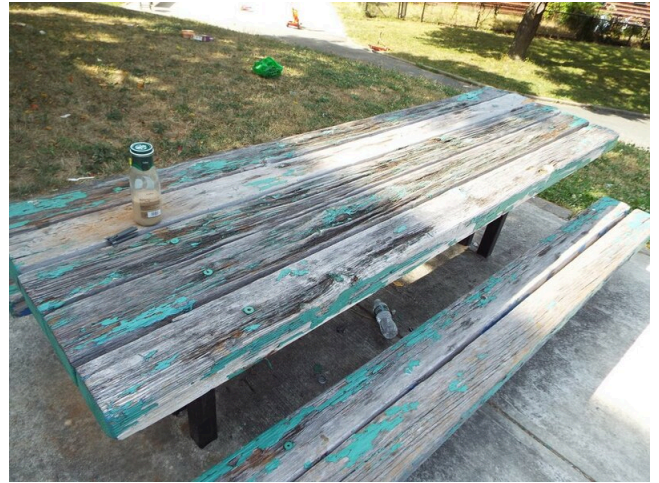
90. Outdoor seating condition - building 17 rear (Non-Critical Repair)
