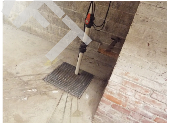
140. Ground water sump pump - building 15
