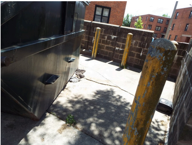
27. Dumpster pad condition - building 7 (Non-Critical Repair)
