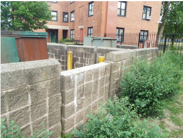
71. Missing dumpster enclosure cap section - building 14-15 (Non-Critical Repair)
