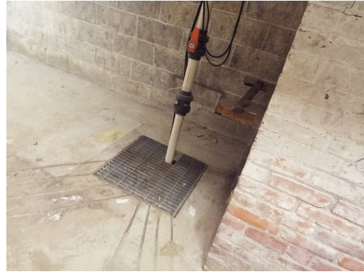
Ground water sump pump - building 15
