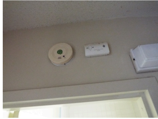
1-bed-1-bath - unit 90D - building 19 - hall smoke and CO2 detectors
