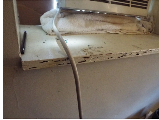
3-bed-1-bath-UFAS - unit 13 - building 4 - termites reported (Non-Critical Repair)
