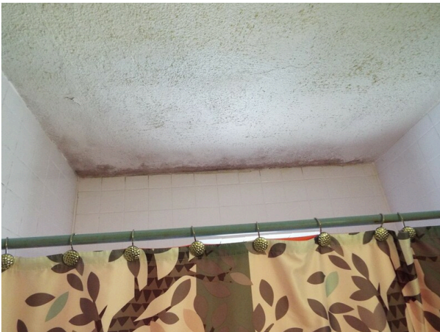
87. 2-bed-1-bath - unit 230D - building 1 - bathroom ceiling mold (Critical Repair)
