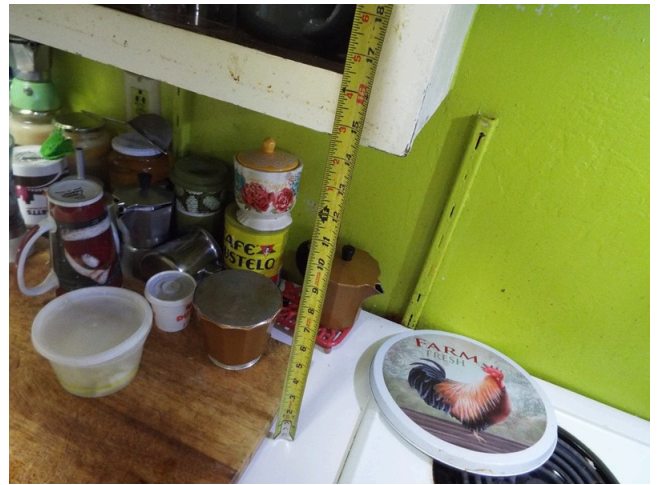
186. UFAS kitchen cabinet shelf exceeds 48 Inch height - unit 53 - building 8
