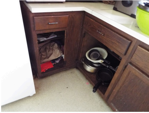
4-bed-2-bath - unit 17 - building 4 - missing kitchen cabinet doors (Non-Critical Repair)
