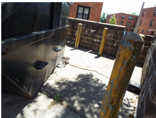
Dumpster pad condition - building 7 (Non-Critical Repair)
