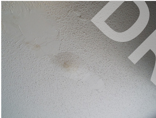
3-bed-1-bath-UFAS - unit 58 - building 8 - kitchen ceiling condition (Non-Critical Repair)
