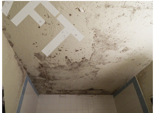
164. 3-bed-1.5-bath-TH - unit 214 - building 3 - bathroom ceiling mold (Critical Repair)
