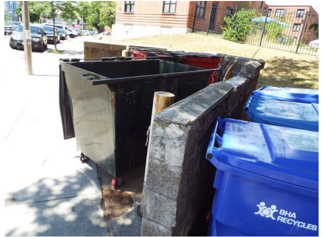
70. Missing dumpster enclosure cap section - building 10 (Non-Critical Repair)
