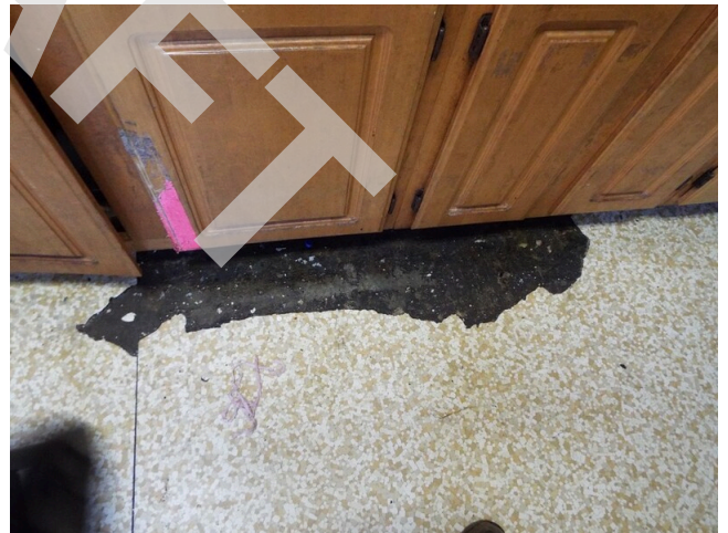
364. 1-bed-1-bath - unit 21A - building 6 - kitchen flooring condition (Non-Critical Repair)
