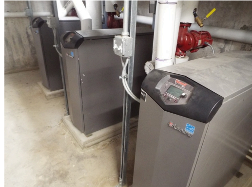
Heating hot water boilers - building 15
