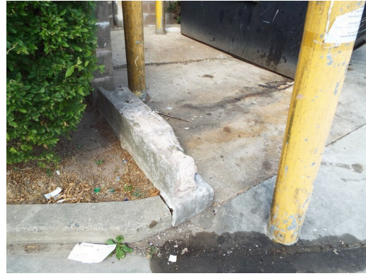
Dumpster wall damage - building 14-17 (Non-Critical Repair)
