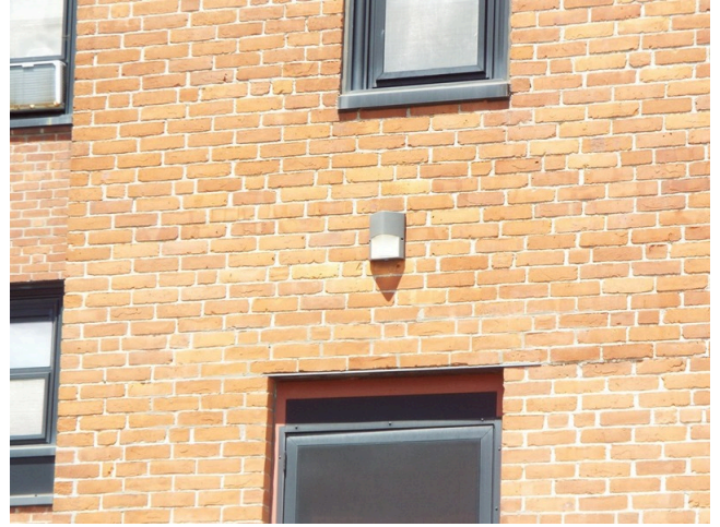
62. Building mounted lighting
