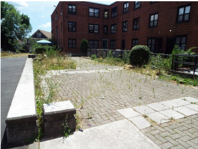
55. Overgrown vegetation - building 7 (Non-Critical Repair)
