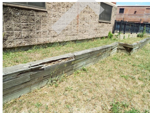
Wood timber retaining wall condition - rear building 9 (Non-Critical Repair)
