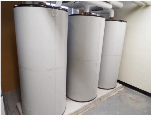
Domestic hot water storage tanks - building 18
