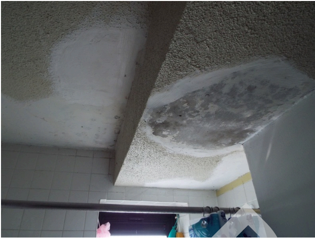
357. 4-bed-2-bath - unit 17 - building 4 - bathroom ceiling mold (Critical Repair)
