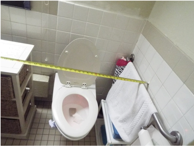
249. UFAS toilet lacks rear grab bar- unit 13 - building 4 (Critical Repair)
