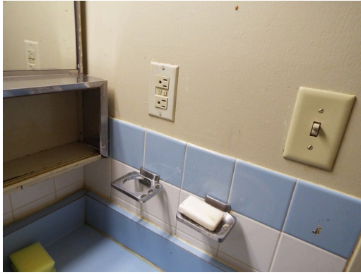
1-bed-1-bath - unit 90D - building 19 - typical bathroom GFCI
