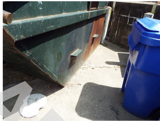
Dumpster pad condition - building 1 (Non-Critical Repair)
