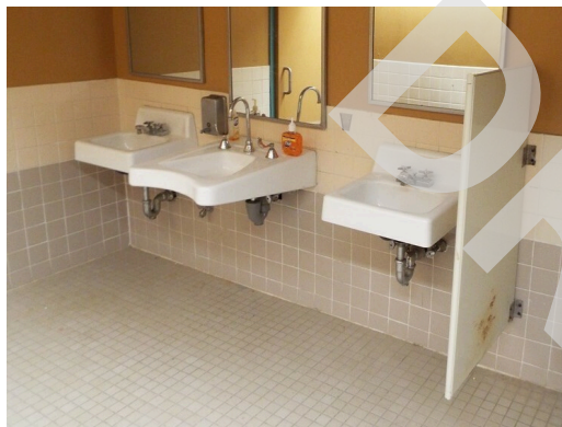
Common area - building 18 - teen center - men's restroom 2 of 3 sinks lack pipe protection (Critical Repair)
