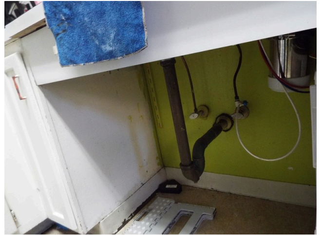
182. UFAS kitchen sink lacks pipe protection - unit 53 - building 8 (Critical Repair)
