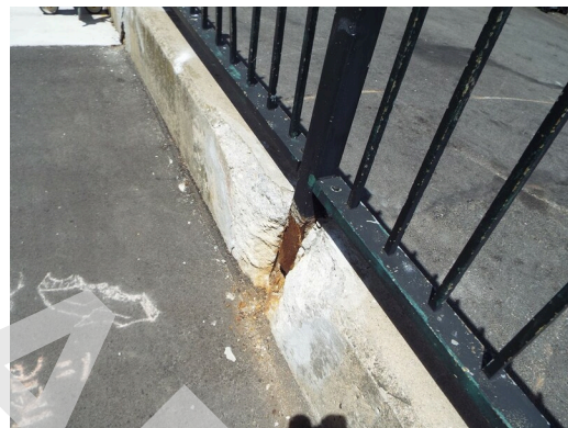
Concrete retaining wall spalling - rear building 12 (Non-Critical Repair)
