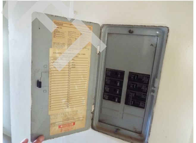
16. 1-bed-1-bath - unit 90D - building 19 - unit electrical panel
