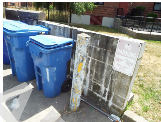
Missing dumpster enclosure cap section - building 1 (Non-Critical Repair)
