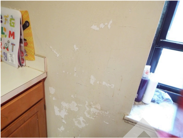
341. 2-bed-1-bath - unit 50E - building 18 - wall paint condition (Non-Critical repair)
