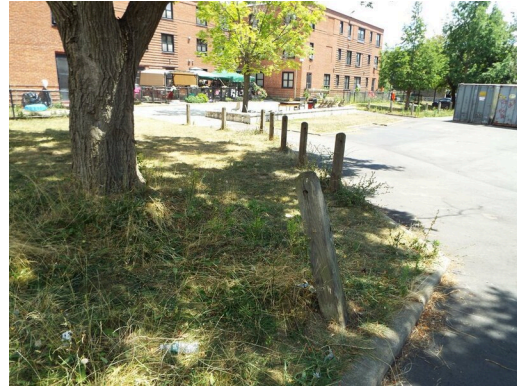
Wood fence post condition - rear buildings 9-12(Non-Critical Repair)
