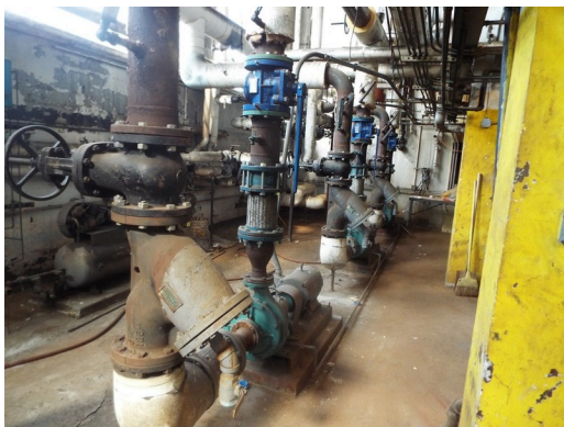
Heating hot water pumps - building 12
