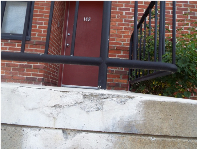
39. Concrete stair spalling - building 16 (Non-Critical Repair)
