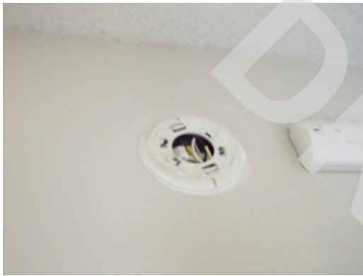
1-bed-1-bath - unit 90D - building 19 - missing smoke detector (Critical Repair)
