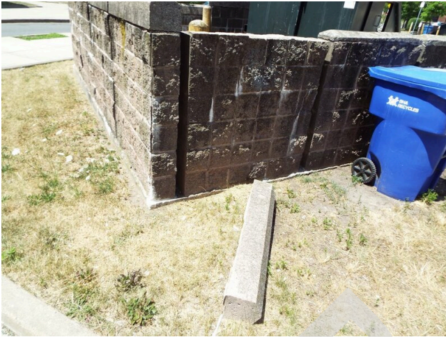
69. Missing dumpster enclosure cap section - building 7 (Non-Critical Repair)
