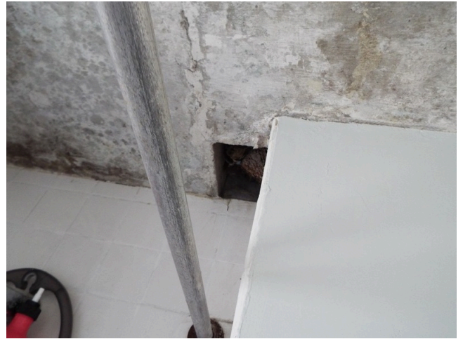
118. 3-bed-1.5-bath-TH - unit 22 - building 17 - bathroom ceiling condition (Critical Repair)
