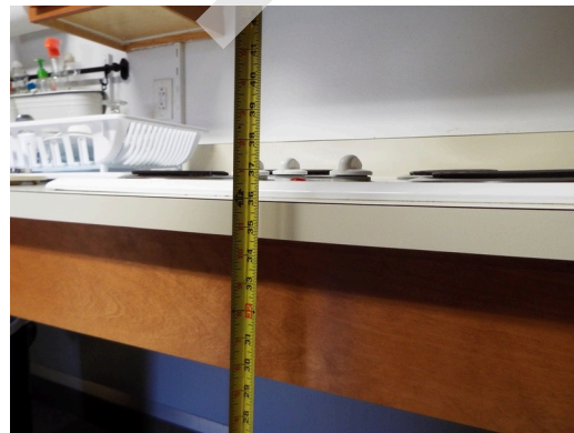
UFAS unit 172 - building 13 - kitchen sink counters exceed 34 inch height (Critical Repair)
