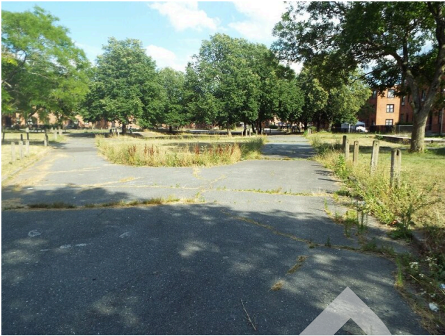
21. Asphalt paving - rear buildings 1 thru 6 (Non-Critical Repair)
