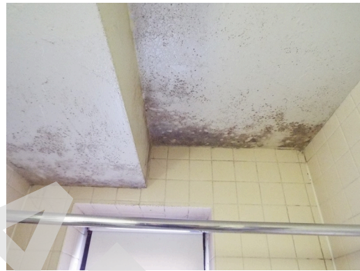
1-bed-1-bath - unit 21A - building 6 - bathroom ceiling mold (Critical Repair)
