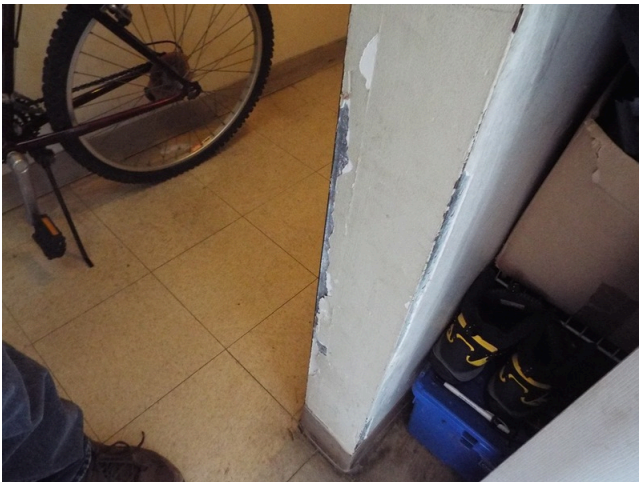
275. 3-bed-1-bath-UFAS - unit 13 - building 4 - wall condition (Non-Critical Repair)
