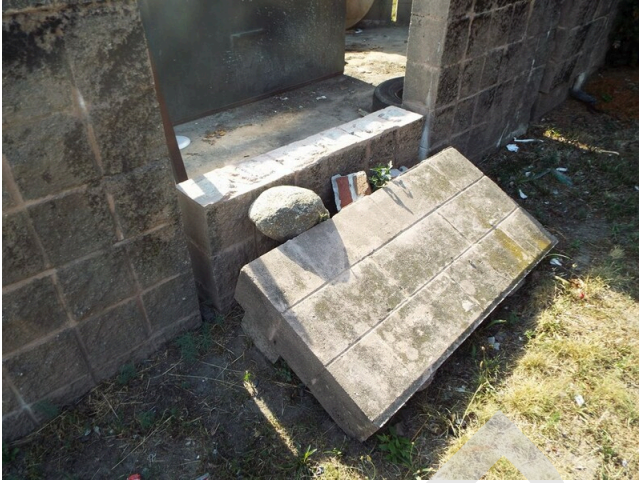
65. Dumpster enclosure wall damage - building 5 (Non-Critical Repair)
