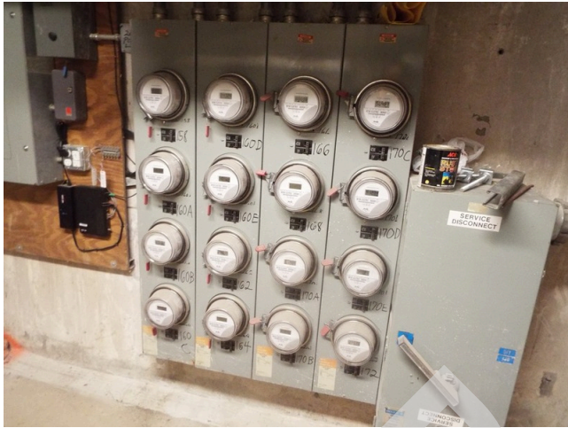
153. Electrical meters - building 15
