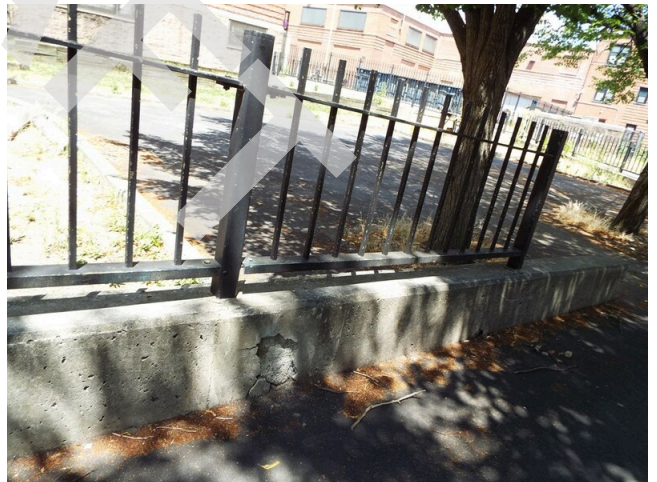
8. Concrete retaining wall spalling - rear building 9 (Non-Critical Repair)
