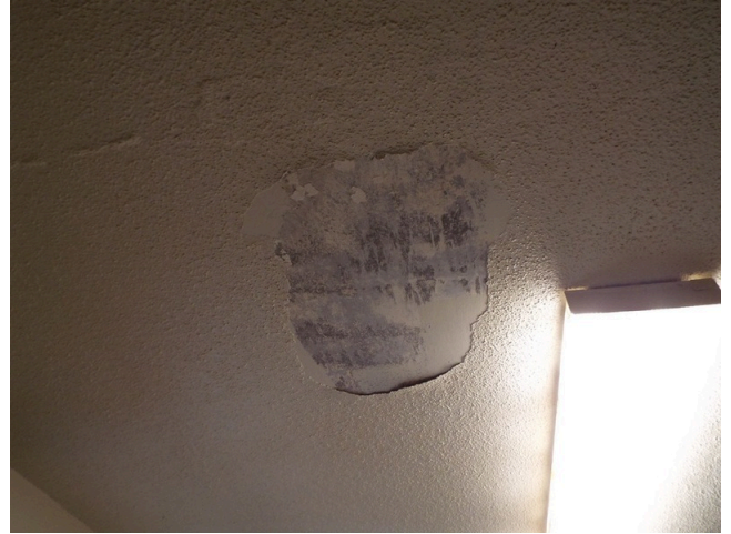
98. 2-bed-1-bath - unit 240A - building 1 - ceiling paint condition (Non-Critical Repair)
