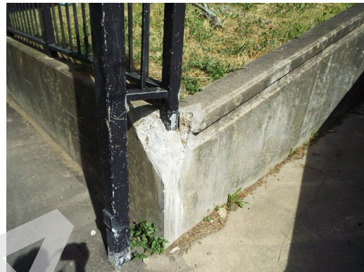
Concrete retaining wall spalling - building 19 (Non-Critical Repair)
