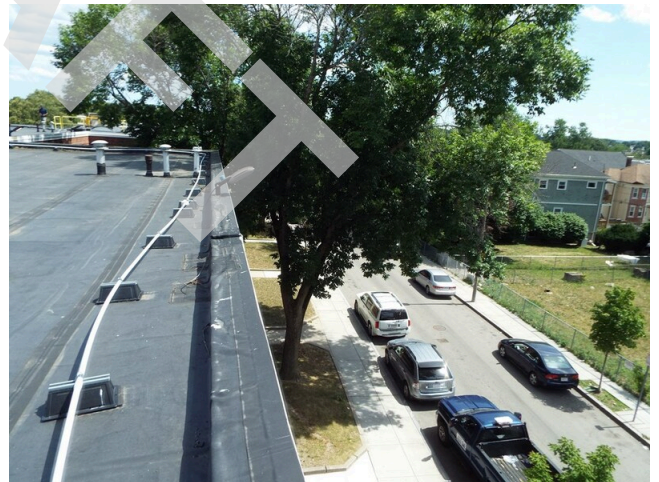
52. Overhanging tree - building 2 (Non-Critical Repair)
