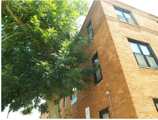
Overhanging tree - building 8 (Non-Critical Repair)
