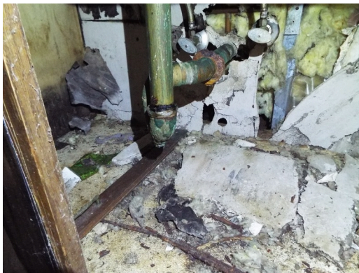
4-bed-2-bath - unit 17 - building 4 wall damage (Non-Critical Repair)
