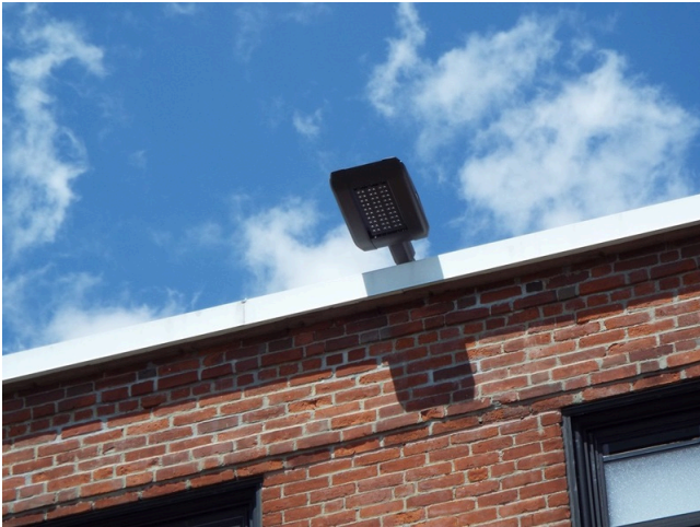
63. Building mounted lighting
