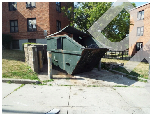
Dumpster pad condition - building 18-19 (Non-Critical Repair)
