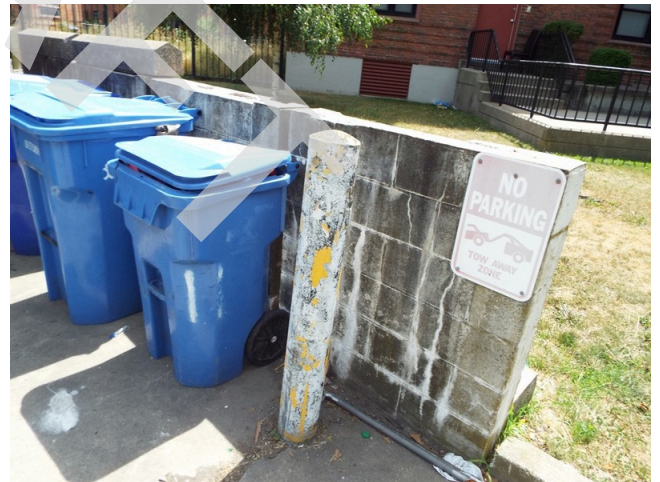
68. Missing dumpster enclosure cap section - building 1 (Non-Critical Repair)
