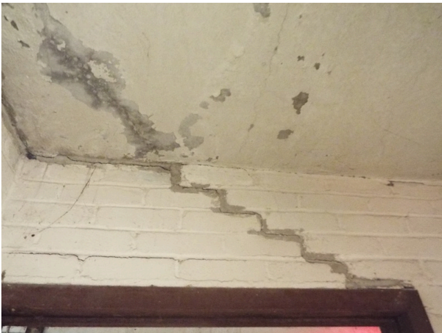
83. Masonry wall cracks - basement building 15 (Non-Critical Repair)
