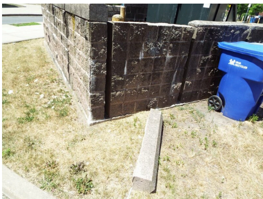
Missing dumpster enclosure cap section - building 7 (Non-Critical Repair)
