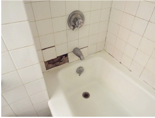
3-bed-1.5 bath - unit 42 - building 17 - bathroom shower tile condition (Non-Critical Repair)
