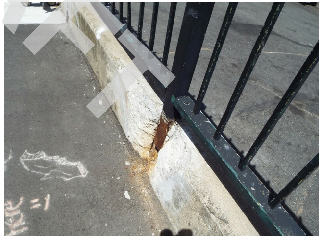
12. Concrete retaining wall spalling - rear building 12 (Non-Critical Repair)
