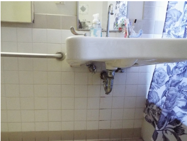
199. UFAS bathroom sink lacks pipe protection - unit 53 - building 8 (Critical Repair)
