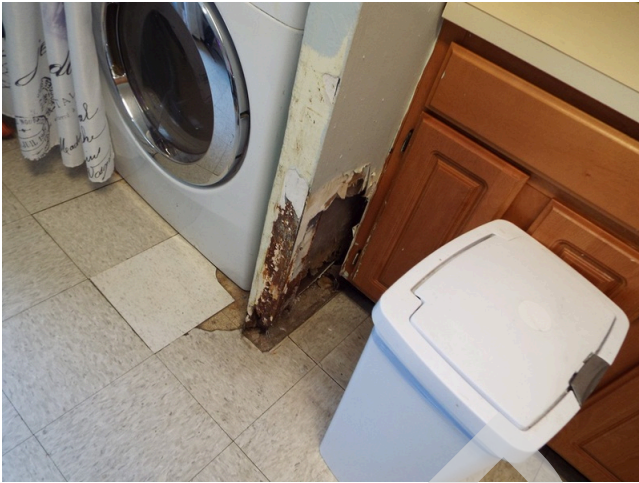
117. 3-bed-1.5-bath-TH - unit 22 - building 17 - washer wall condition (Non-Critical Repair)
