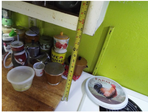
UFAS kitchen cabinet shelf exceeds 48 inch height - unit 13 - building 4 (Critical Repair)
