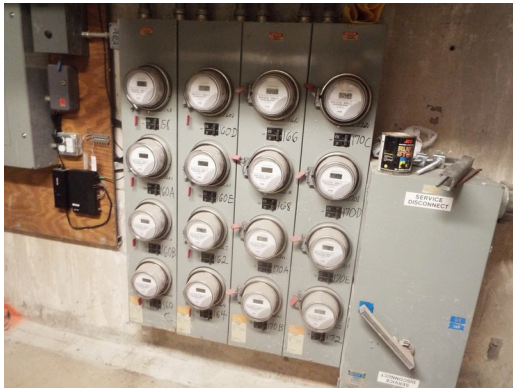
Electrical meters - building 15
