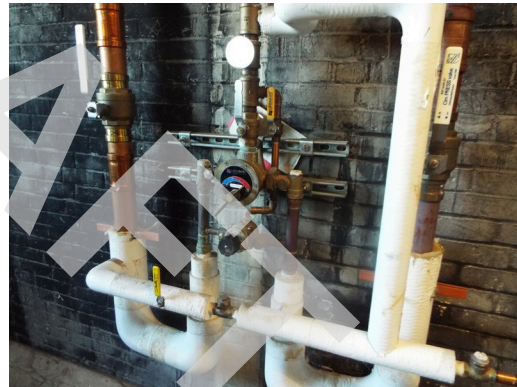
Domestic hot water mixing valves - building 12 (2)
