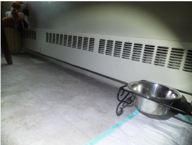
79. 2-bed-1-bath - unit 160C - building 15 - baseboard heating unit
