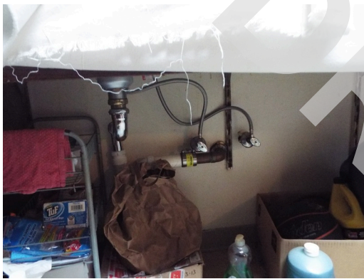
UFAS kitchen sink lacks pipe protection - unit 13 - building 4
