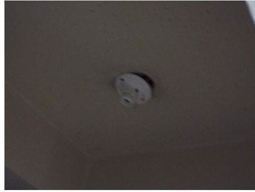
2-bed-1-bath - unit 50G - building 18 - loose light fixture (Critical Repair)
