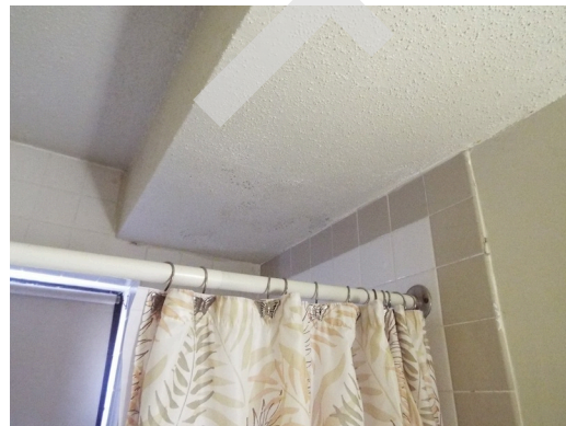
3-bed-1-bath-UFAS - unit 13 - building 4 - bathroom ceiling mold (Critical Repair)
