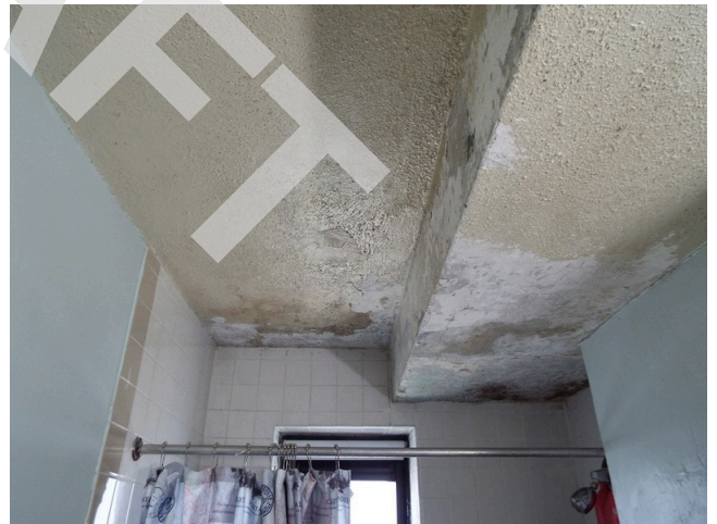
120. 3-bed-1.5-bath-TH - unit 22 - building 17 - bathroom ceiling condition (Critical Repair)
