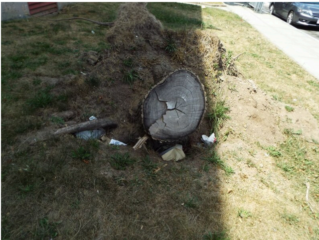
51. Hole at stump - building 4 (Critical Repair)
