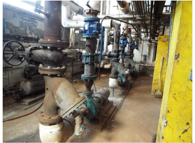
150. Heating hot water pumps - building 12
