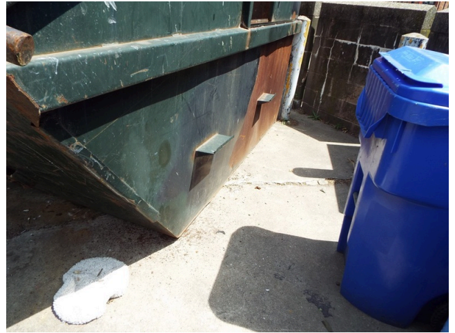
26. Dumpster pad condition - building 1 (Non-Critical Repair)
