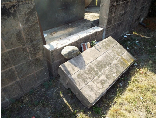
Dumpster enclosure wall damage - building 5 (Non-Critical Repair)
