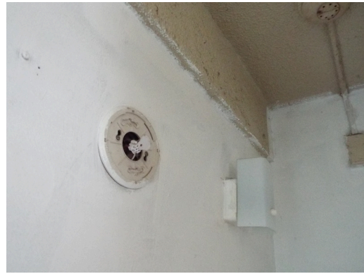
4-bed-2-bath - unit 17 - building 4 - missing smoke detector (Critical Repair)
