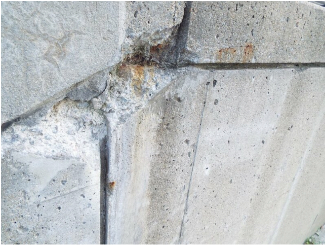
38. Concrete stair spalling - building 15 (Non-Critical Repair)
