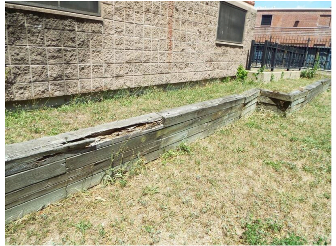
14. Wood timber retaining wall condition - rear building 9 (Non-Critical Repair)
