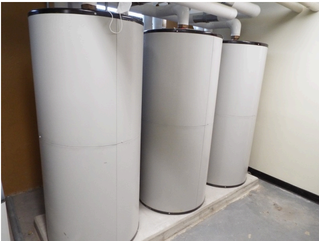
143. Domestic hot water storage tanks - building 18
