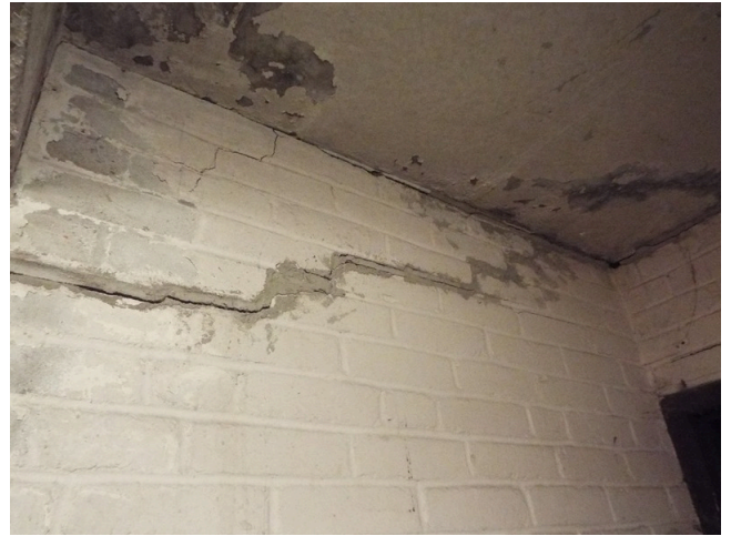
82. Masonry wall cracks - basement building 15 (Non-Critical Repair)
