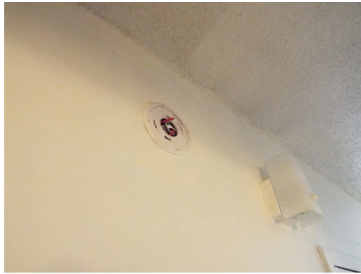
2-bed-1-bath - unit 82 - building 7 UFAS - missing smoke detector (Critical Repair)
