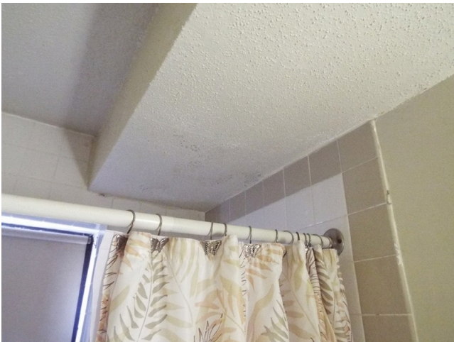
267. 3-bed-1-bath-UFAS - unit 13 - building 4 - bathroom ceiling mold (Critical Repair)
