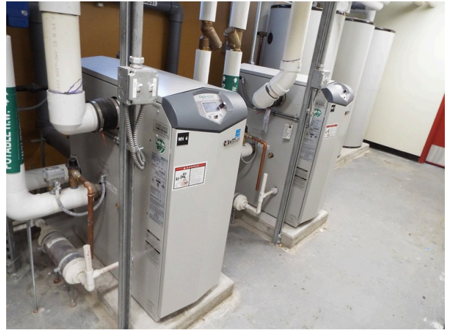
142. Domestic hot water boilers - building 18
