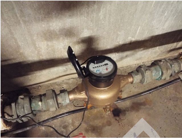
141. Water meter - building 15
