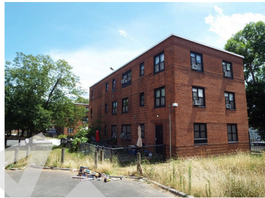
Overgrown vegetation - building 10 (Non-Critical Repair)
