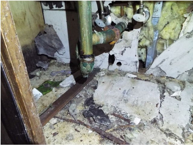
353. 4-bed-2-bath - unit 17 - building 4 wall damage (Non-Critical Repair)
