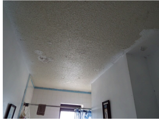
4-bed-2-bath - unit 17 - building 4 - ceiling condition (Non-Critical Repair)
