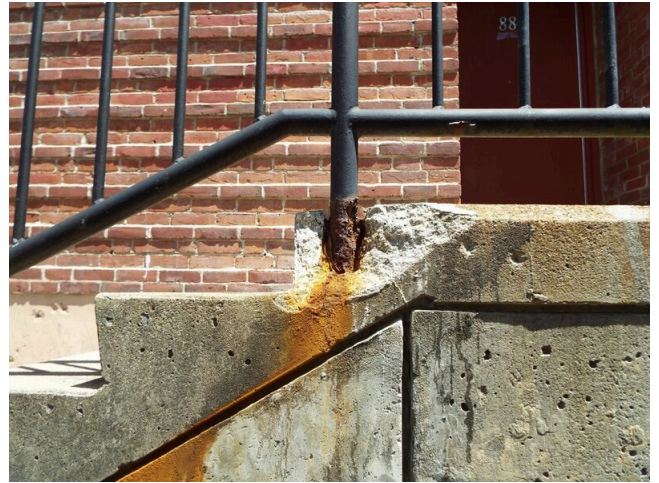
42. Concrete step spalling and handrail post base condition - building 7 unit 88 (Non-Critical Repair)
