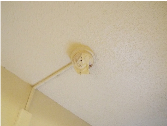
335. 5-bed-2-bath-TH - unit 190A - building 14 - disabled smoke detector (Critical Repair)
