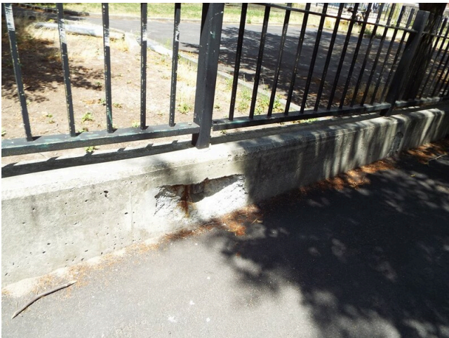
7. Concrete retaining wall spalling - rear building 9 (Non-Critical Repair)
