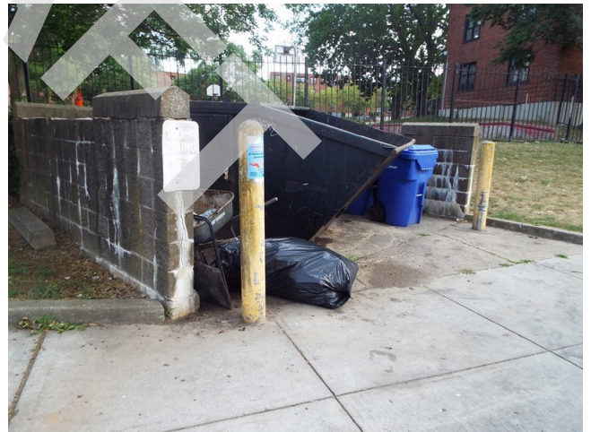
72. Missing dumpster enclosure cap section - building 15-16 (Non-Critical Repair)
