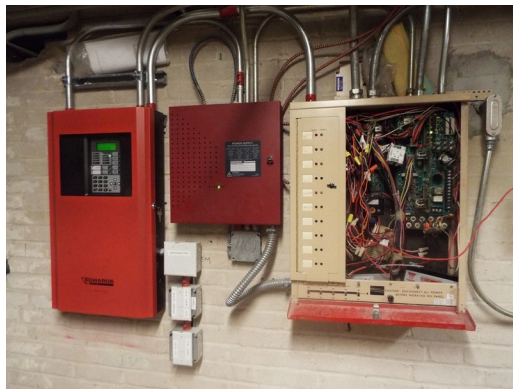
Fire alarm control panel - building 15
