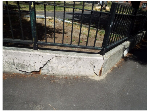
Concrete retaining wall spalling - rear building 9 (Non-Critical Repair)
