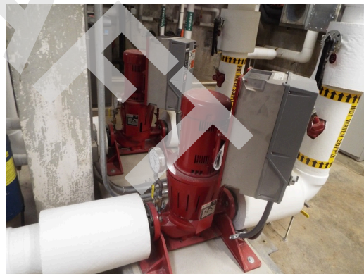
Heating hot water pumps - building 15
