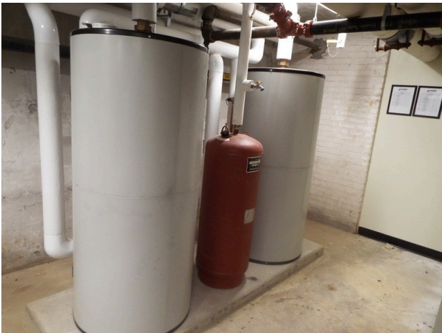
139. Domestic hot water storage tanks - building 15
