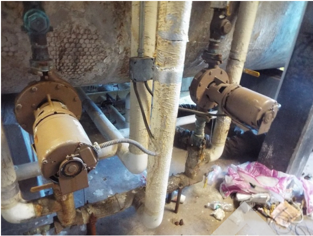
137. Domestic hot water circulation pumps - building 12
