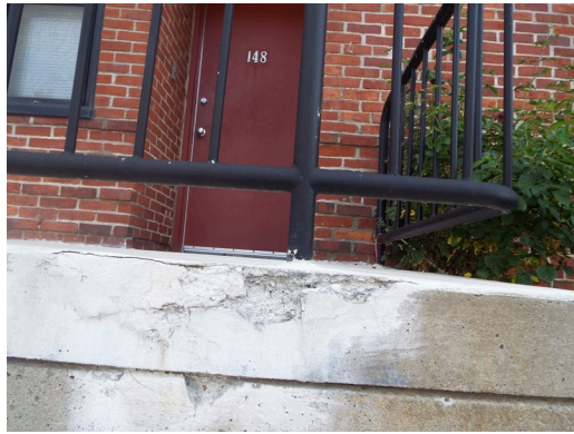
Concrete stair spalling - building 16 (Non-Critical Repair)
