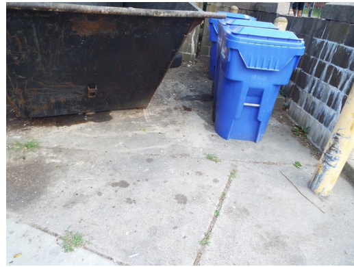
Dumpster pad condition - building 15-16 (Non-Critical Repair)
