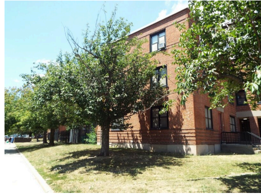
Overhanging tree - building 12 (Non-Critical Repair)
