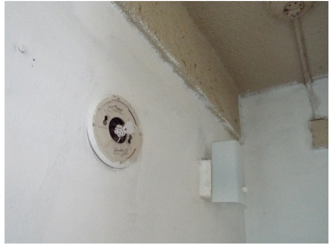
358. 4-bed-2-bath - unit 17 - building 4 - missing smoke detector (Critical Repair)
