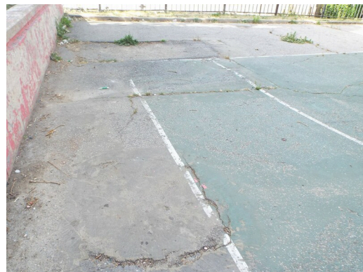
Basketball court surface condition (Non-Critical Repair)
