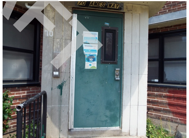
92. Building entry door condition - building 7 (Non-Critical Repair)
